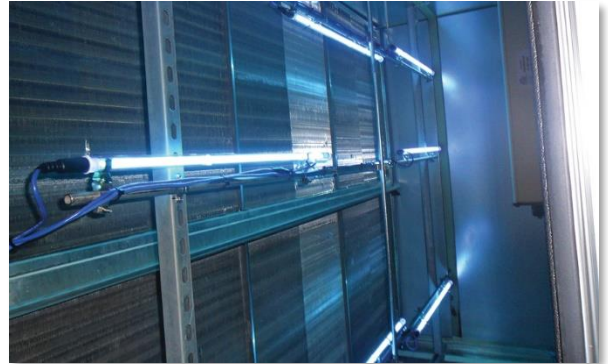
Figure 8- UVGI in an HVAC system
