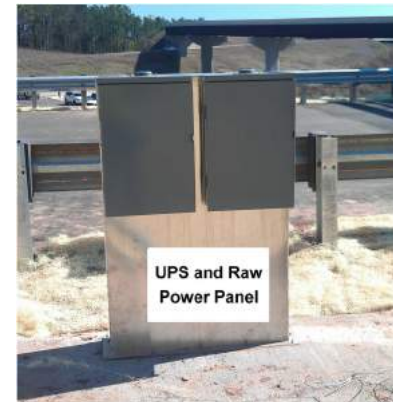
Pad Typical "B" Zone Electronics, AVI and ITS/DMS Cabinets w/ Power Panel N.T.S.
