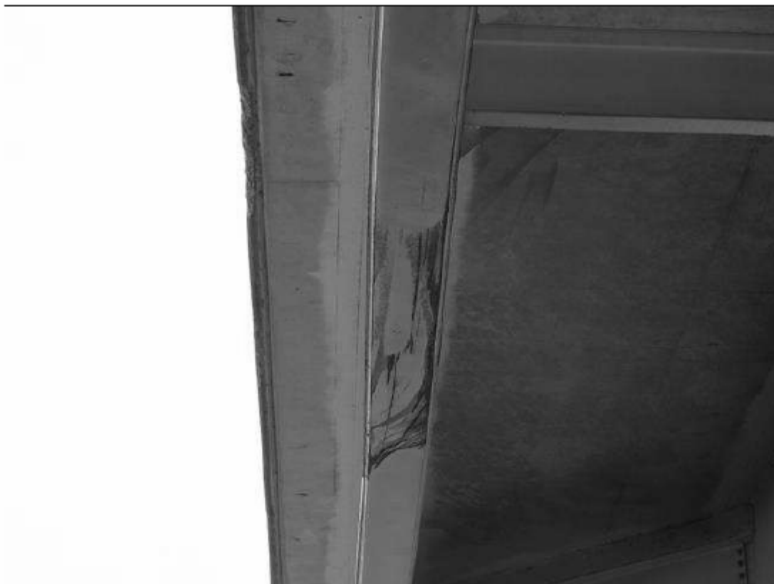
Span 2 Beam 1: IMPACT DAMAGE WITH 1/2" OF DISTORTION IN WEB AND BOTTOM FLANGE
