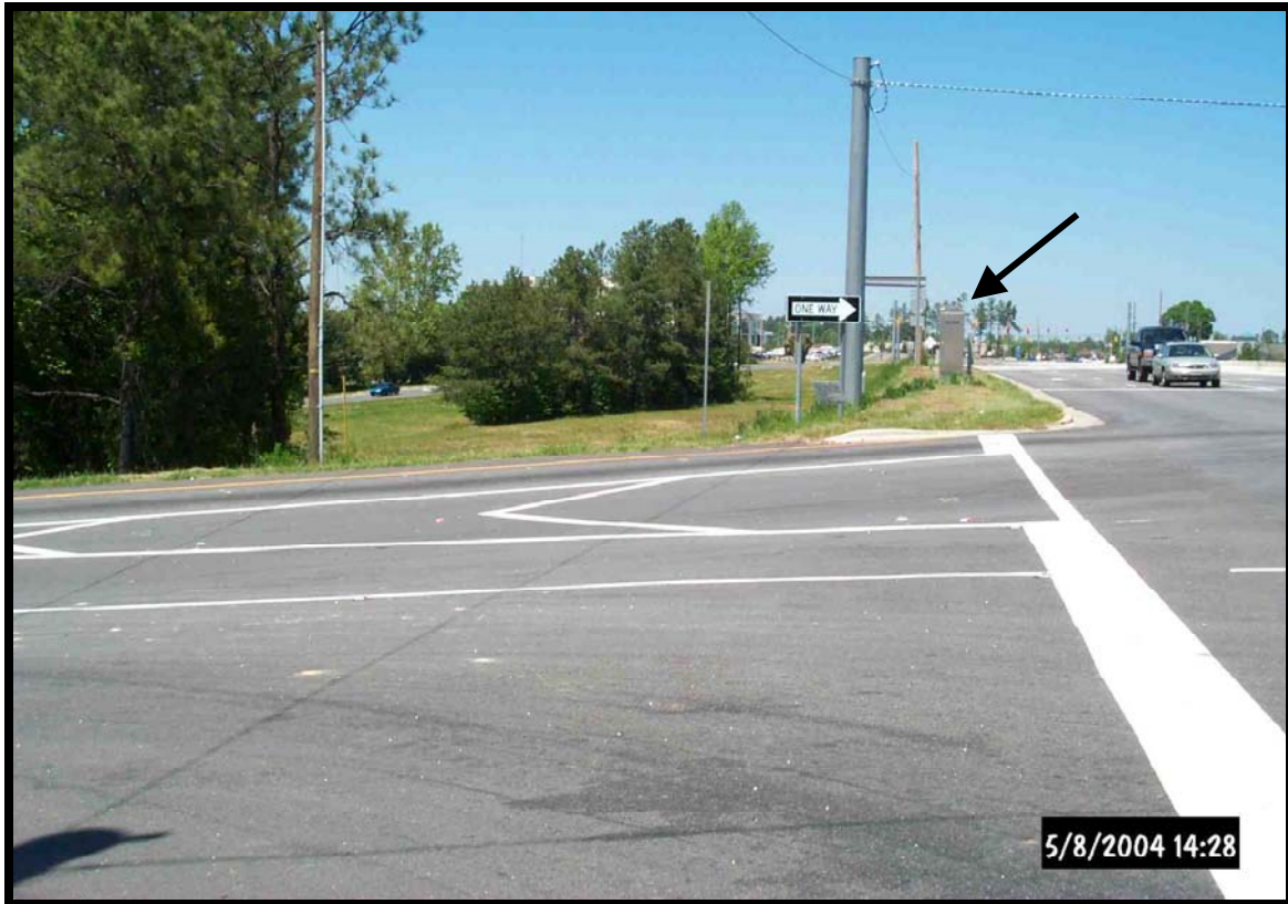
Signal control box and electric power meter located on berm at Ramp B intersection with SR 1128. This box will have to be relocated if sidewalk is constructed in the future. The electric power meter is located on a pedestal between the signal control box and the curb and gutter.
