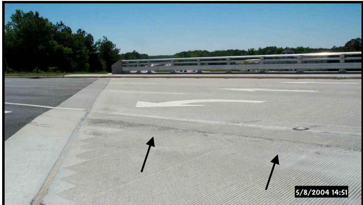
Ridge in bridge deck due to unequal deflections during staged deck construction
