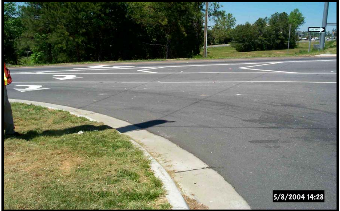
Steep rollover at Ramp B-SR 1128 intersection
