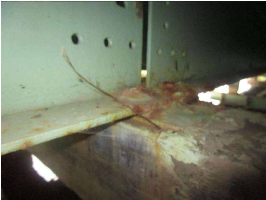
Span 5 Beam 10 - Near Bearing: ANCHOR BOLT COMPLETELY CORRODED, PAR
