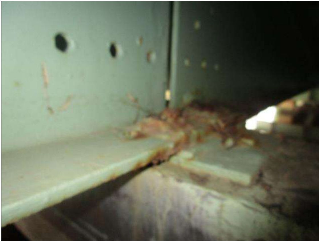
Span 5 Beam 11 - Near Bearing: ANCHOR BOLT COMPLETELY CORRODED, PAR
