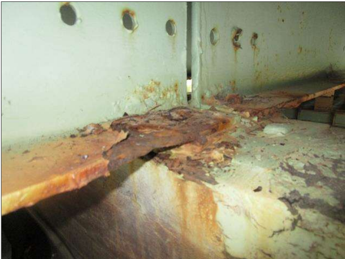
Span 5 Beam 2 - Near Bearing: ANCHOR BOLT COMPLETELY CORRODED, PAR
