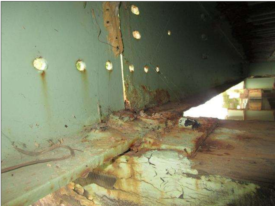
Span 5 Beam 12 - Near Bearing: ANCHOR BOLT COMPLETELY CORRODED, PAR
