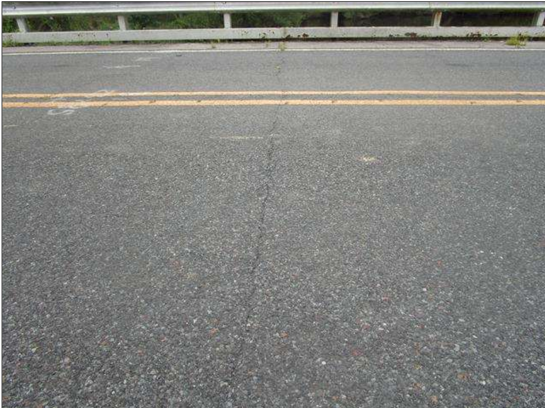
Span 3 Wearing Surface: ALONG BENT 2, FULL WIDTH X UP TO 1/16IN WIDE TRANSVERSE CRACK IN THE ASPHALT WEARING SURFACE
