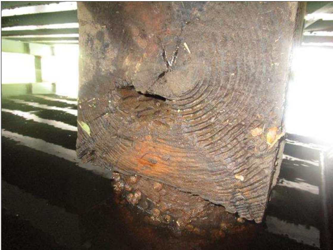
Bent 2 Cap 2: NORTH END OF THE SUB CAP AT PILE 3 WATERLINE, 3IN DIAMETER X 4IN DEEP DECAYED AREA, PAR
