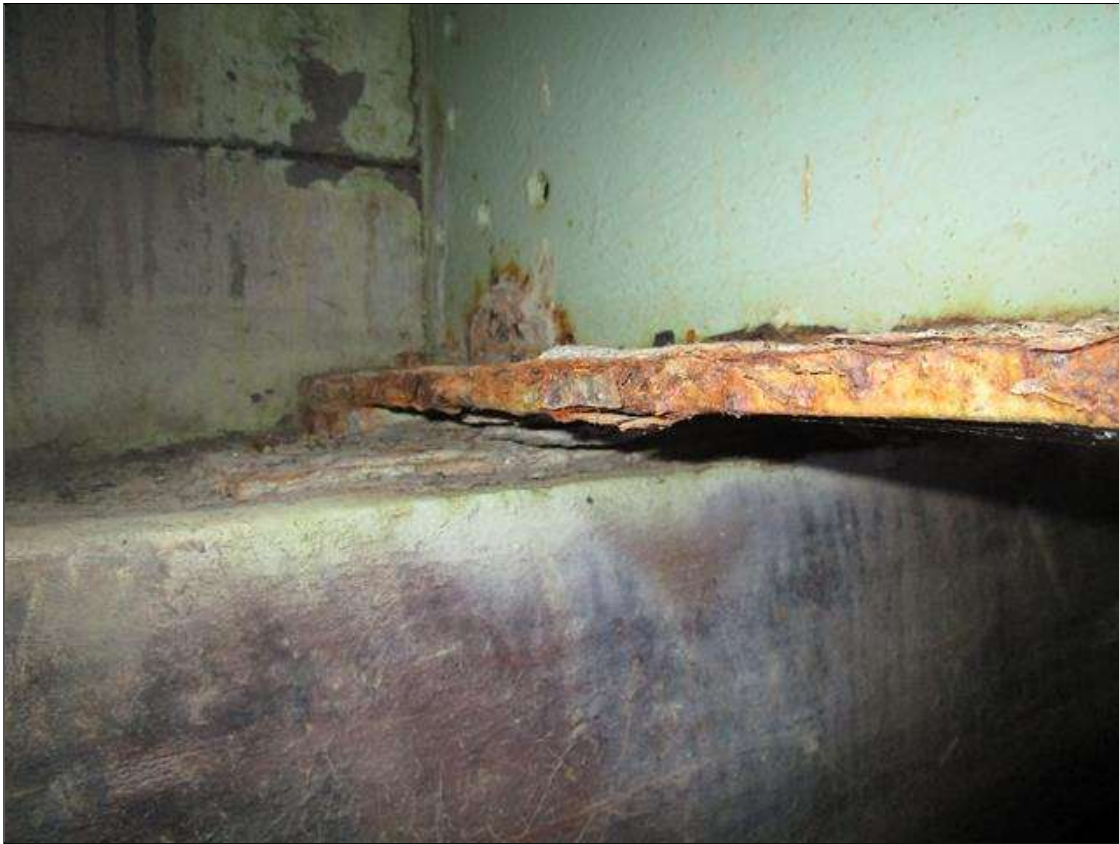
Span 1 Beam 5: SPAN 1, AT END BENT 1, INTERMITTENT FULL LENGTH AREA OF SECTION LOSS DOWN TO 3/8IN REMAINING IN BOTTOM FLANGE, PAR
