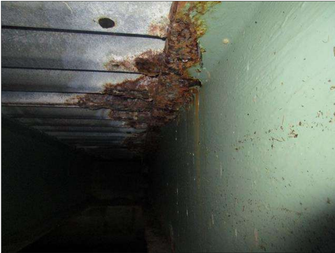
Span 5 Beam 9: TOP FLANGE, AT END BENT 2, 12FT LONG AREA OF SECTION LOSS DOWN TO KNIFE'S EDGE, PAR
