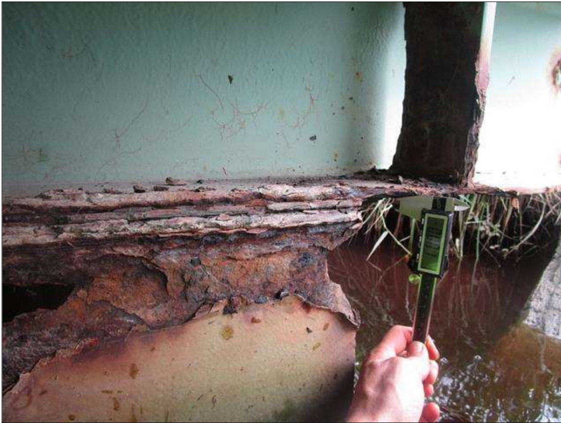
Bent 5 Cap 1: AT BEAM 6, 1/2IN WIDE X 100% SECTION LOSS OF BOTTOM FLANGE, PAR
