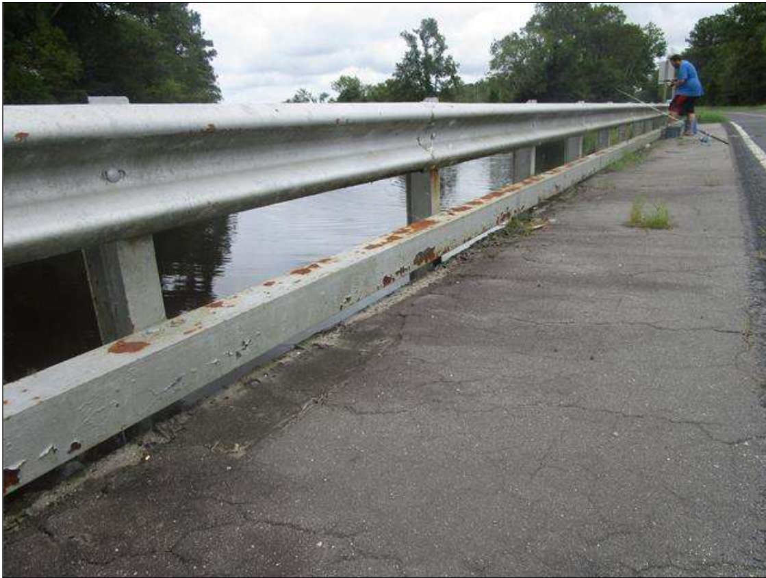
Span 3 Left Bridge Rail: INTERMITTENT FULL LENGTH X 4IN WIDE SURFACE RUST ON THE NORTH CURB
