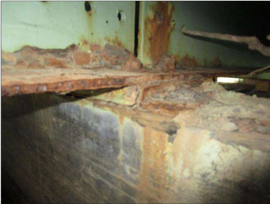
Span 5 Beam 7 - Near Bearing: 1/4IN SECTION LOSS. 3/8IN REMAINING, PAR
