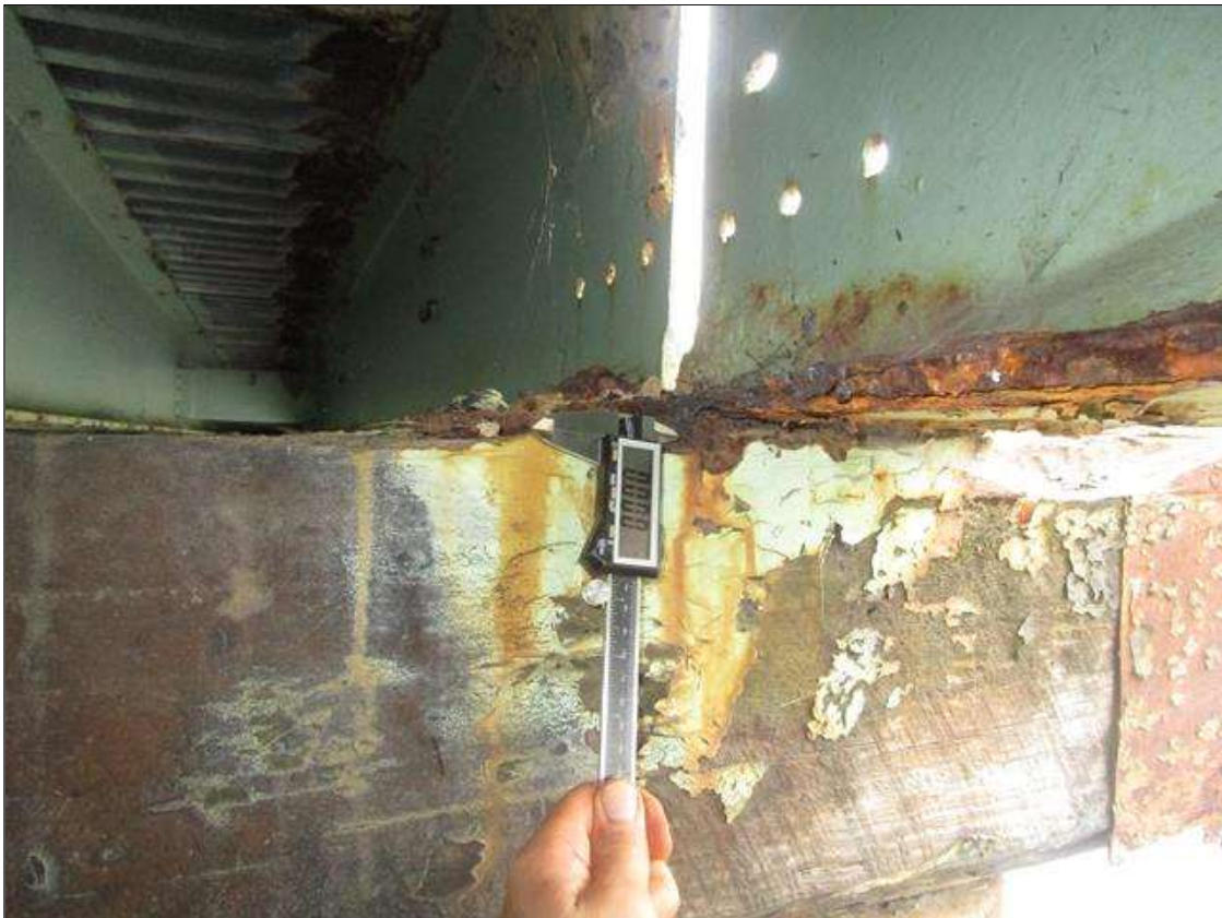
Span 3 Beam 12: SPAN 4, AT BENT 4, 1FT LONG X 2IN X 100% AREA OF SECTION LOSS IN BOTTOM FLANGE, PAR
