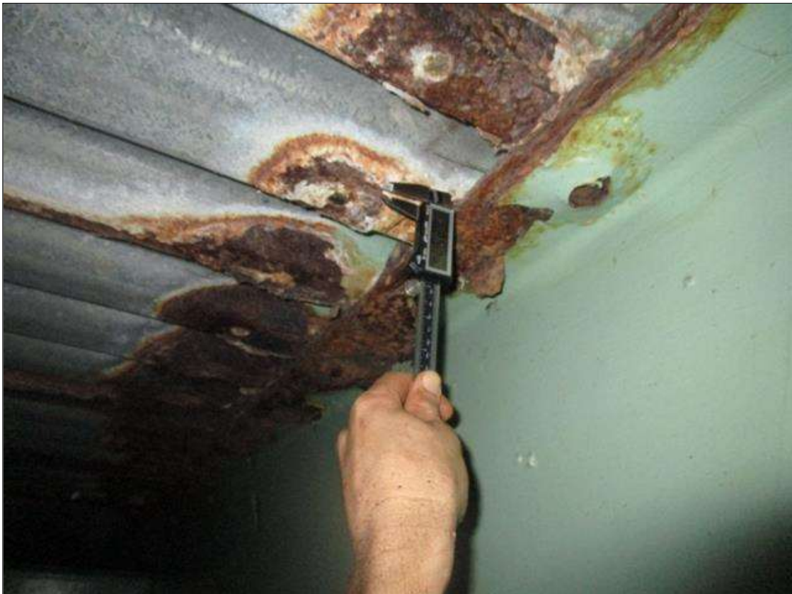
Span 3 Beam 9: SPAN 3, AT BENT 3, 9FT AREA OF SECTION LOSS IN TOP FLANGE DOWN TO 0.249IN REMAINING TOP FLANGE, PAR
