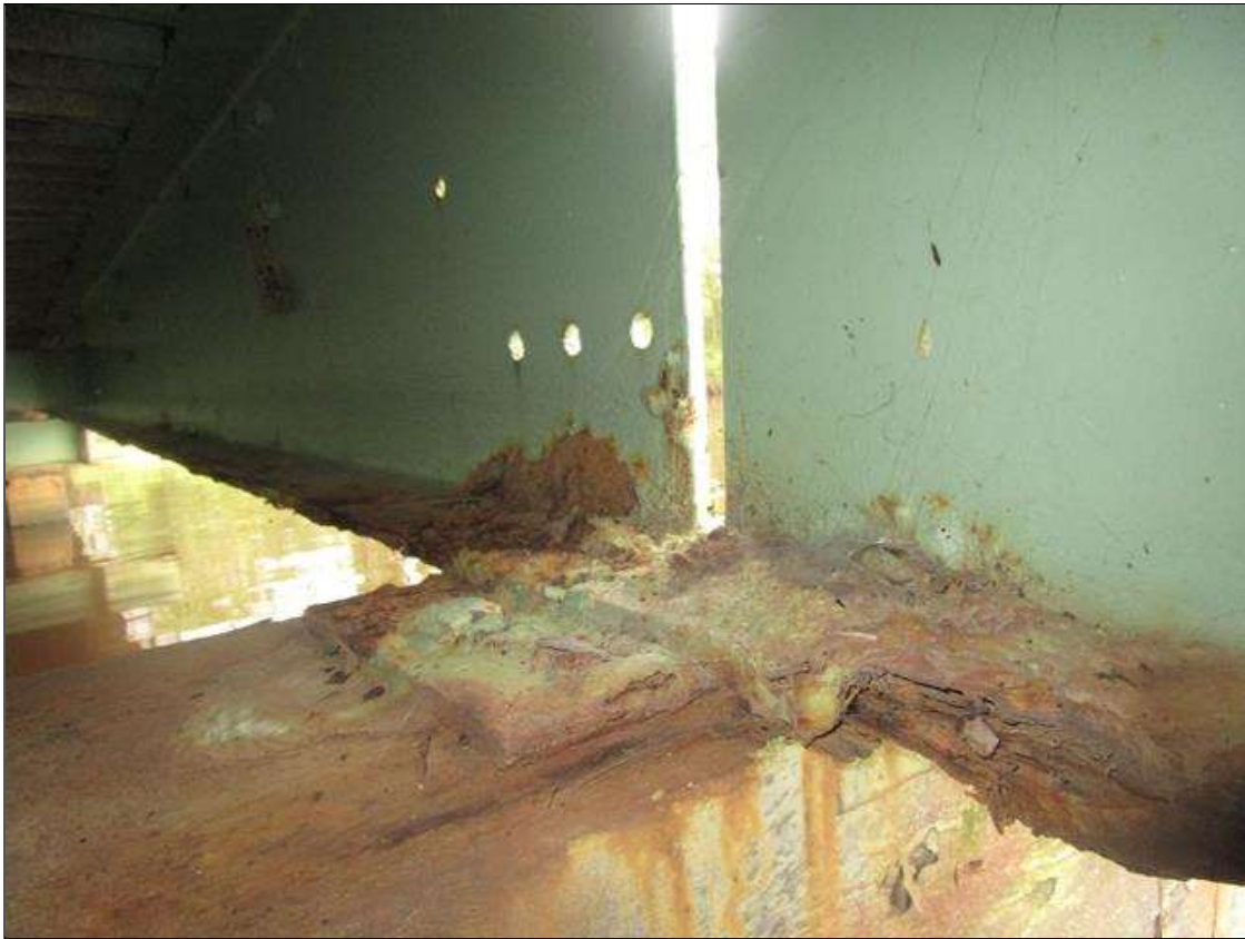
Span 5 Beam 1 - Near Bearing: ANCHOR BOLT COMPLETELY CORRODED, PAR
