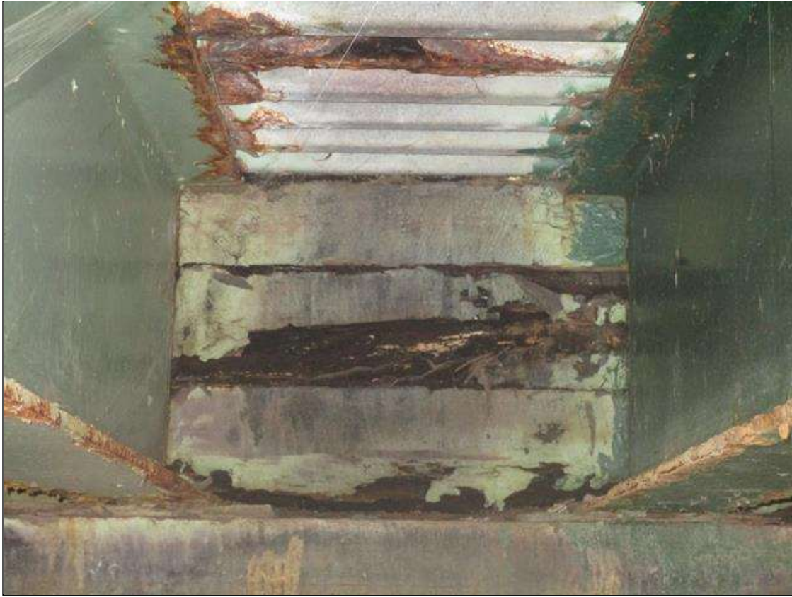
End Bent 1 Abutment: 5'-0" LONG X 8" HIGH X 1" DEEP AREA OF DECAY IN THE BULKHEAD IN BAYS 1 TO 3. (BAY 2 SHOWN)
