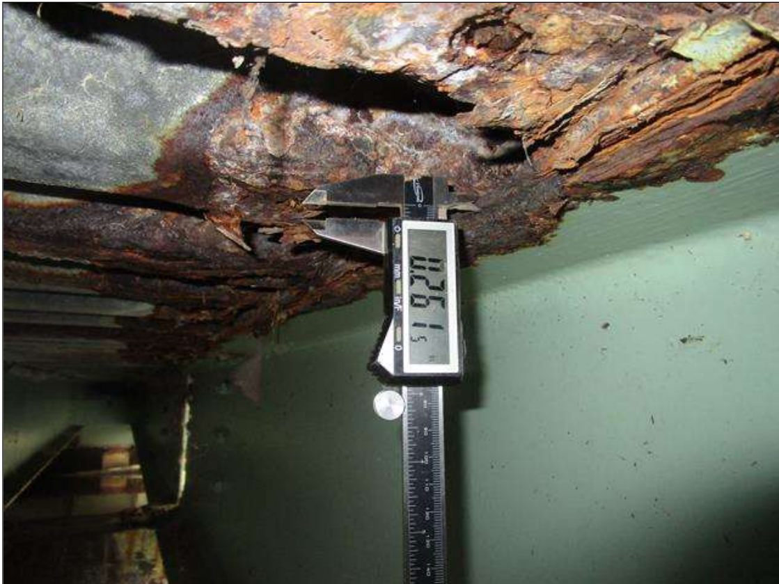
Span 3 Beam 12: SPAN 4, INTERMITTENT FULL LENGTH AREA OF SECTION LOSS DOWN TO 0.261IN REMAINING IN TOP FLANGE, PAR
