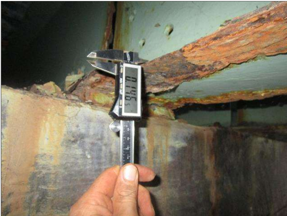
Span 3 Beam 8: SPAN 4, AT BENT 4, 3FT AREA OF SECTION LOSS DOWN TO 0.146IN REMAINING IN BOTTOM FLANGE, PAR
