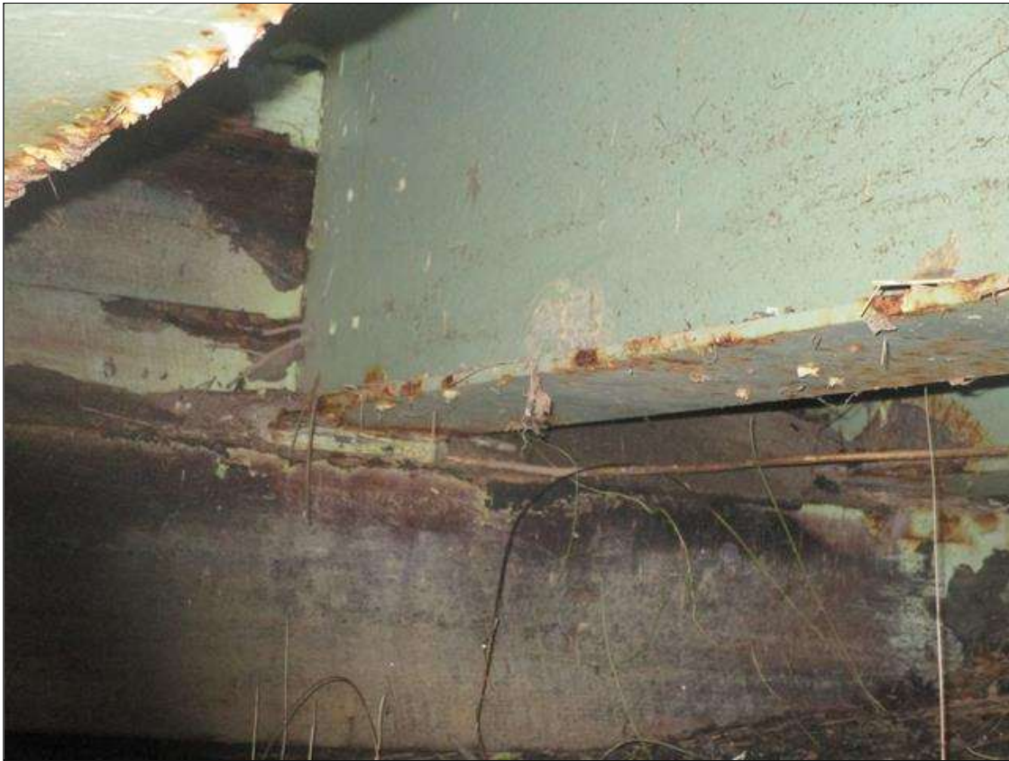
Span 5 Beam 11: SPAN 6, AT END BENT 2, 1FT AREA OF SECTION LOSS DOWN TO 5/16IN REMAINING IN BOTTOM FLANGE, PAR
