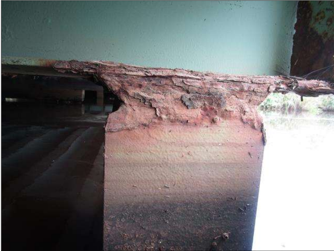
Bent 3 Pile 6: 2IN LONG X 1IN WIDE X 100% SECTION LOSS OF BOTH EDGES AT BOTH FLANGES AT TOP OF PILE. 1/8IN SECTION LOSS IN TOP PLATE, PAR
