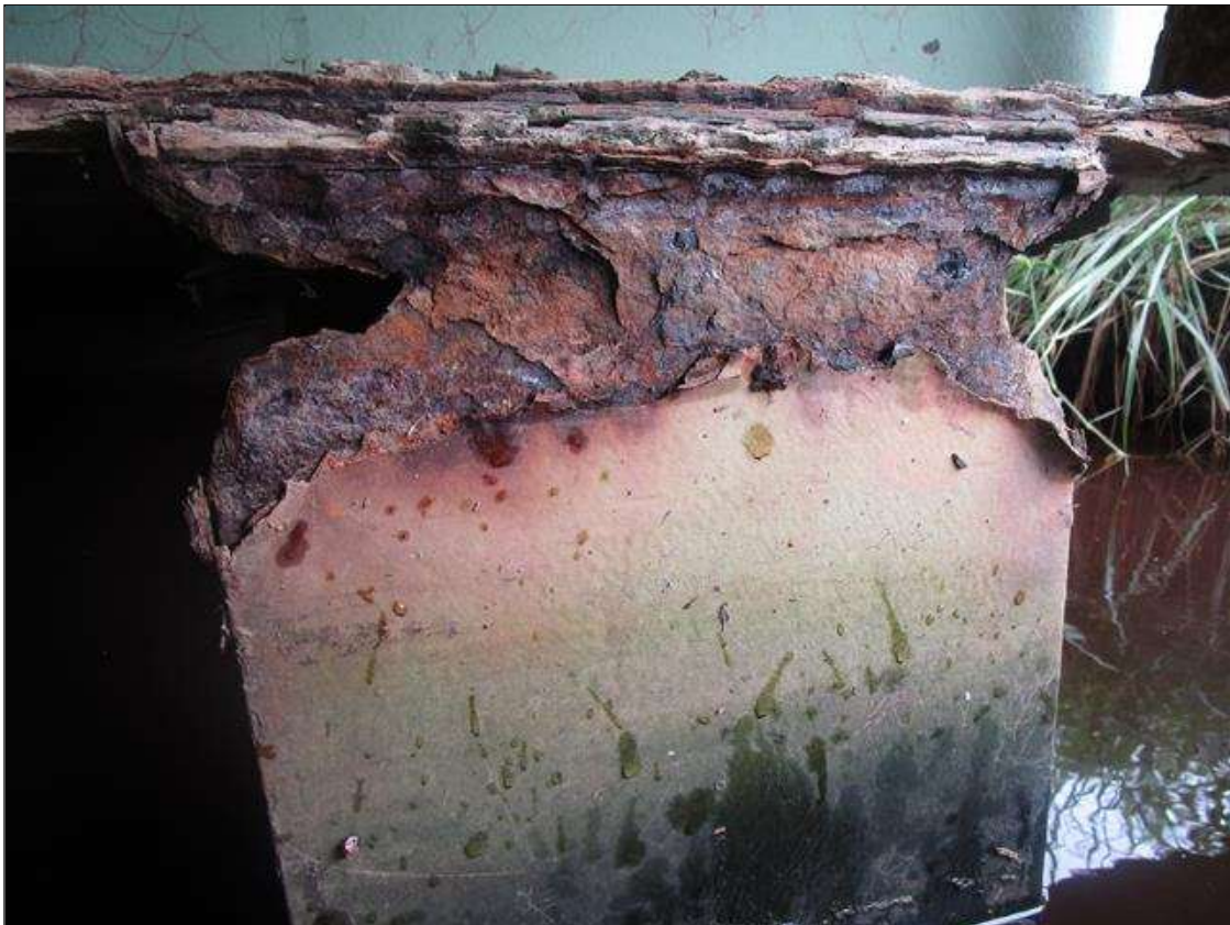
Bent 5 Pile 6: 2IN LONG X 2IN WIDE X 100% SECTION LOSS OF BOTH EDGES AT BOTH FLANGES AT TOP OF PILE. 1/8IN SECTION LOSS IN TOP PLATE, PAR
