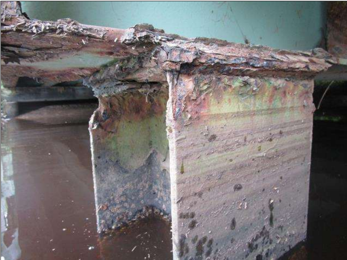
Bent 5 Pile 1: 2IN LONG X 1IN WIDE X 100% SECTION LOSS OF BOTH EDGES AT BOTH FLANGES AT TOP OF PILE. 1/8IN SECTION LOSS IN TOP PLATE, PAR
