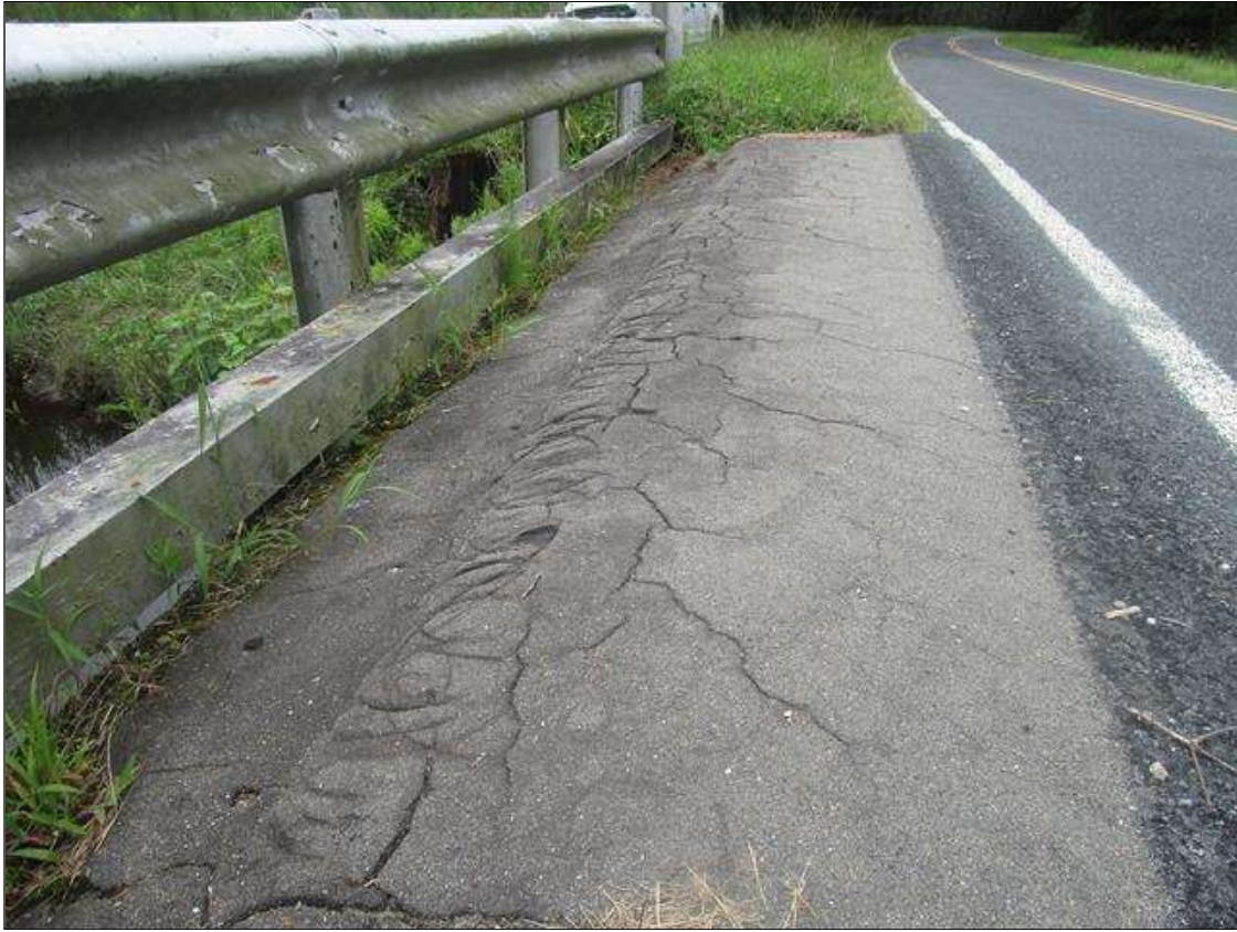
Span 1 Wearing Surface: FULL LENGTH X 4FT WIDE MAP CRACKING UP TO 1/4IN WIDE ALONG THE RIGHT SHOULDER
