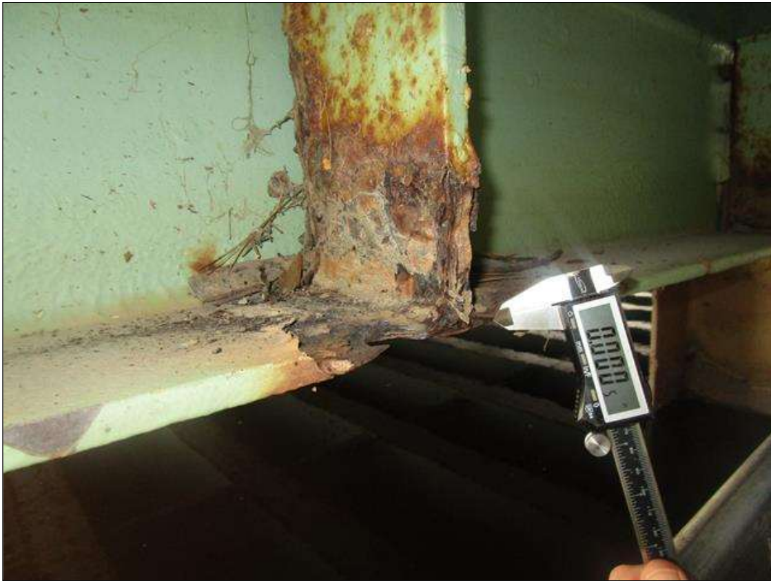
Bent 3 Cap 1: AT BEAM 2, 1IN WIDE X 100% SECTION LOSS, PAR
