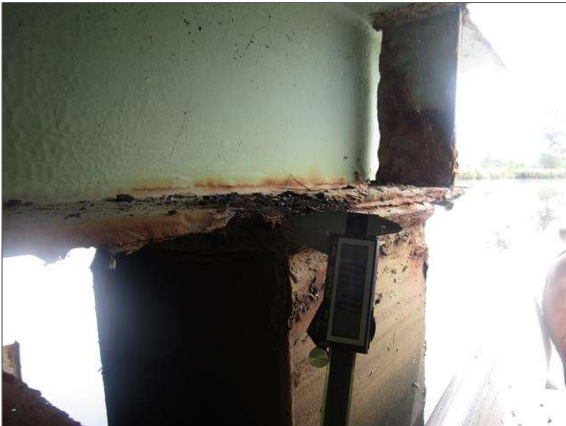
Bent 1 Cap 1: AT BEAMS 11-12 AND PILE 6, 1IN WIDE X 100% SECTION LOSS IN BOTTOM FLANGE, PAR
