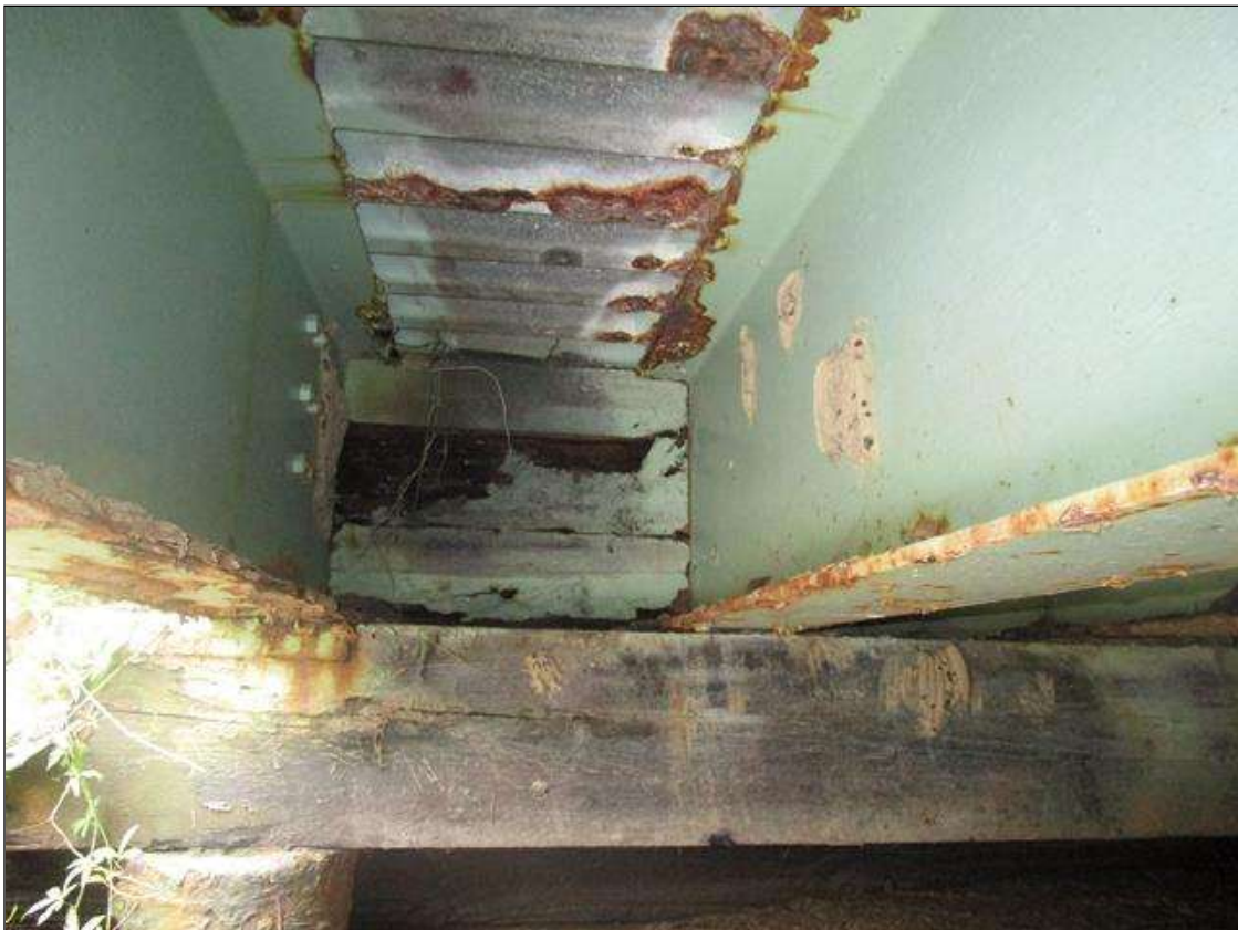
End Bent 2 Abutment: BULKHEAD IN BAY 1, 2'-0" LONG X 8" HIGH X 1" DEEP AREA OF DECAY
