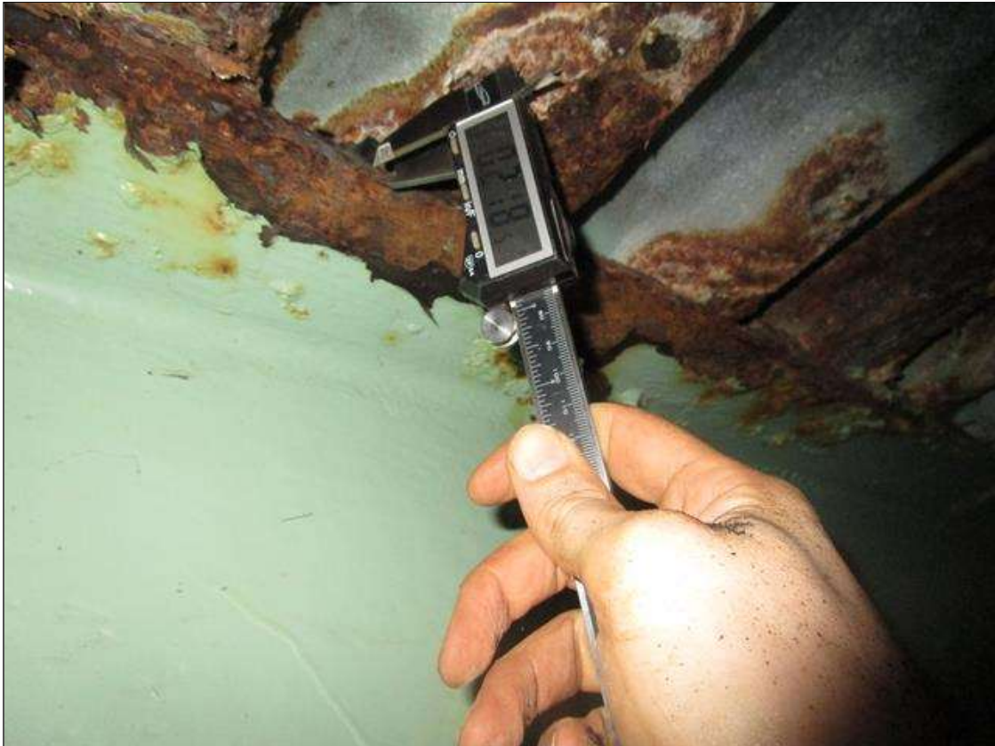
Span 5 Beam 8: SPAN 6, 3FT FROM BENT 5, SECTION LOSS IN TOP FLANGE DOWN TO 0.278IN REMAINING, PAR
