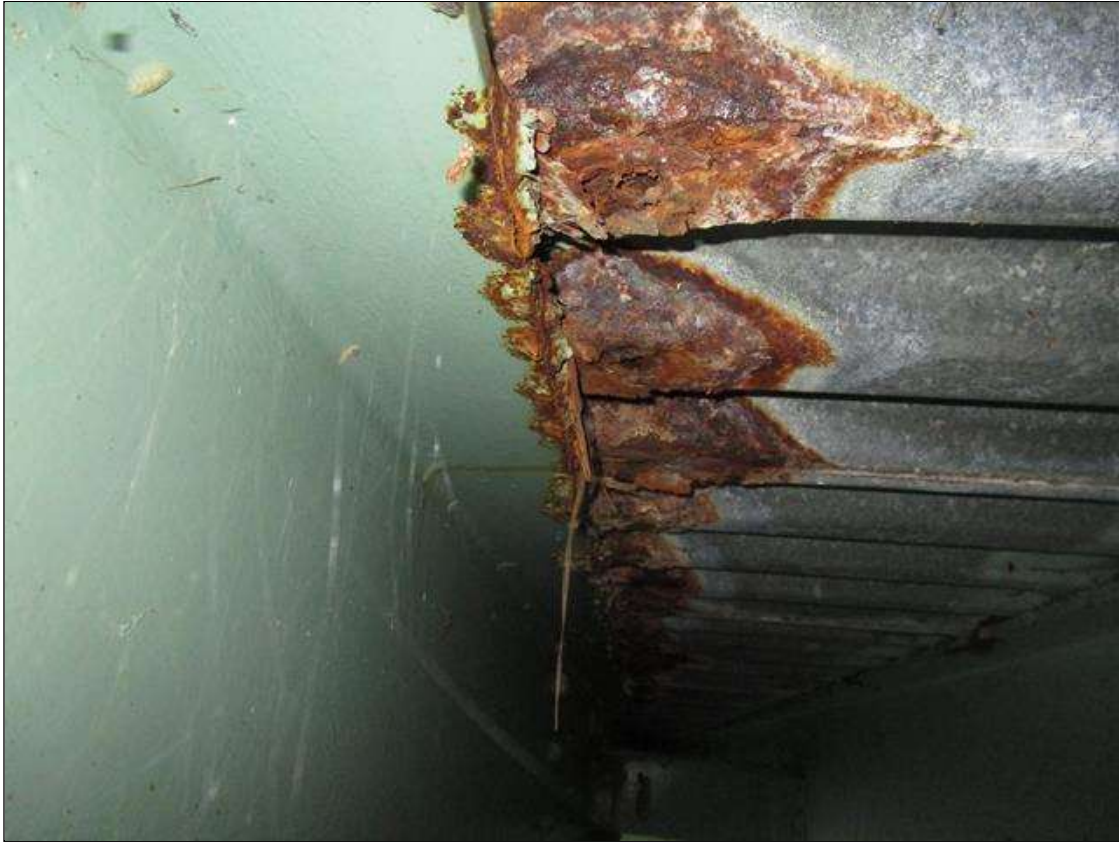
Span 2 Deck: BAY 11, 20FT X 6IN AREA OF CORROSION WITH 25% SECTION LOSS, PAR
