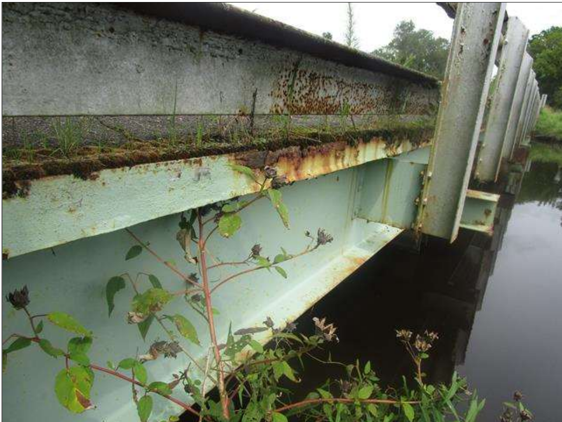
Span 1 Deck: NORTH AND SOUTH DECK FASCIA ANGLES, FULL LENGTH X FULL WIDTH X FULL HEIGHT AREA OF DELAMINATED STEEL ONSET OF SECTION LOSS
