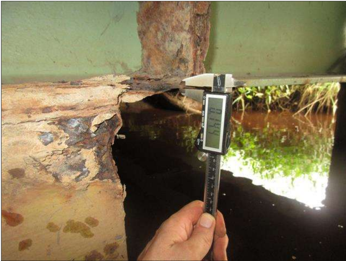
Bent 5 Cap 1: AT BEAM 10, SECTION LOSS IN BOTTOM FLANGE DOWN TO 0.144IN REMAINING, PAR
