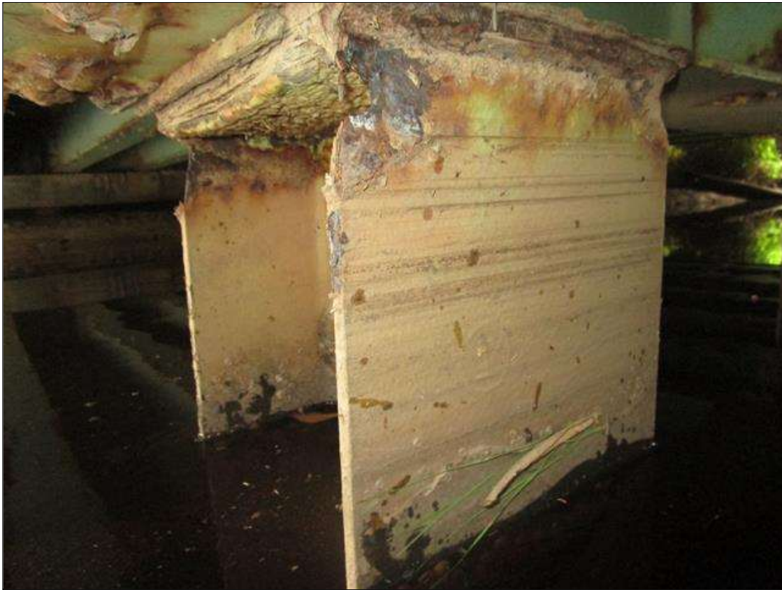
Bent 5 Pile 2: 2IN LONG X 1IN WIDE X 100% SECTION LOSS OF BOTH EDGES AT BOTH FLANGES AT TOP OF PILE. 1/8IN SECTION LOSS IN TOP PLATE, PAR
