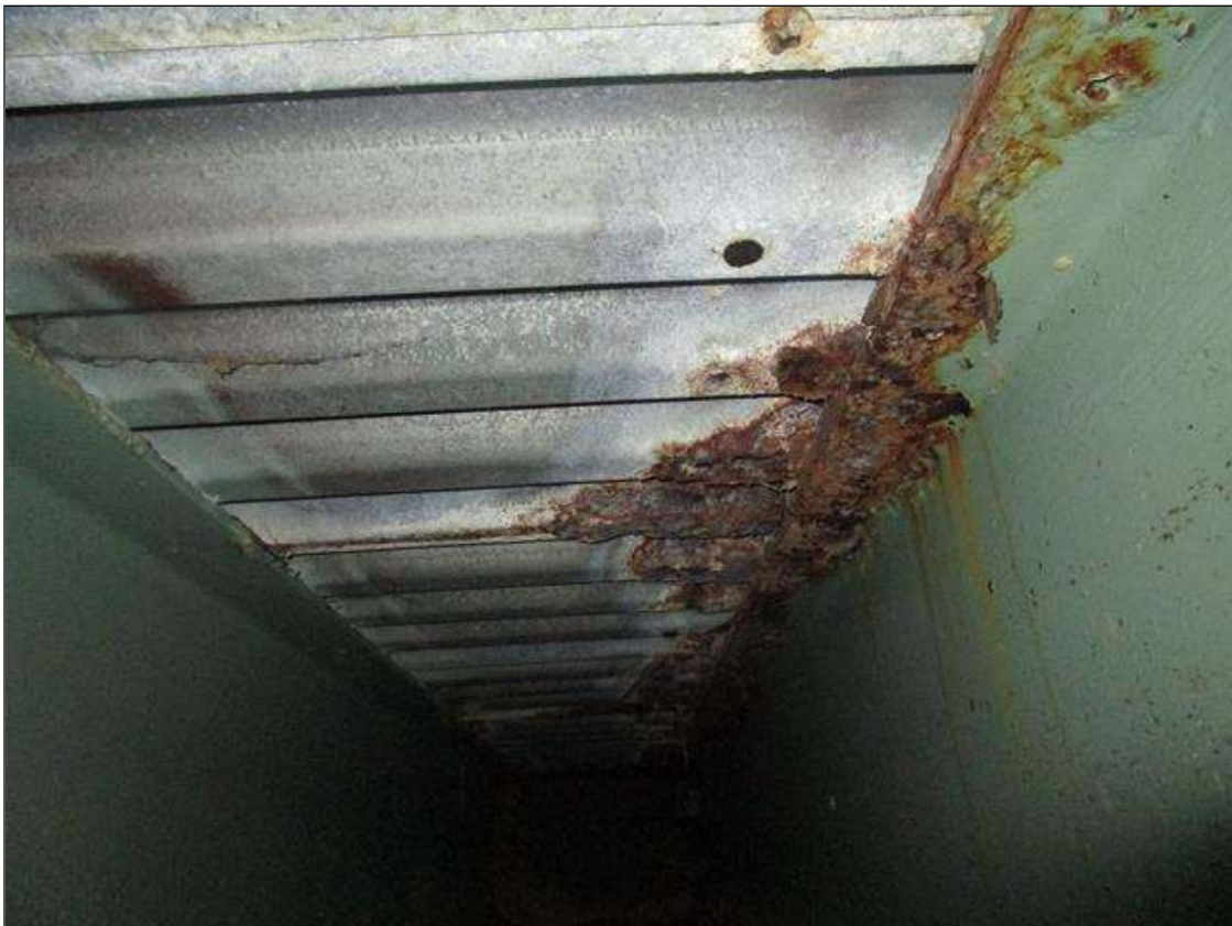
Span 6 Deck: BAY 8 AT END BENT 2, 8FT X 1FT AREA WITH 40% SECTION LOSS, PAR
