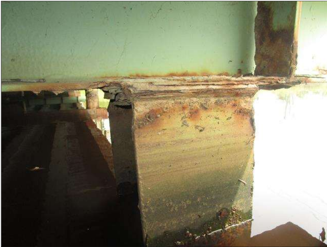
Bent 1 Pile 6: 2IN LONG X 1IN WIDE X 100% SECTION LOSS OF BOTH EDGES AT BOTH FLANGES AT TOP OF PILE. 1/8IN SECTION LOSS IN TOP PLATE, PAR
