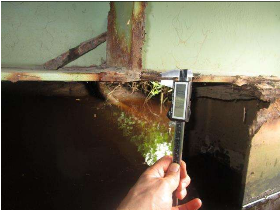
Bent 5 Cap 1: AT BEAM 11, SECTION LOSS IN BOTTOM FLANGE DOWN TO 0.18IN REMAINING, PAR
