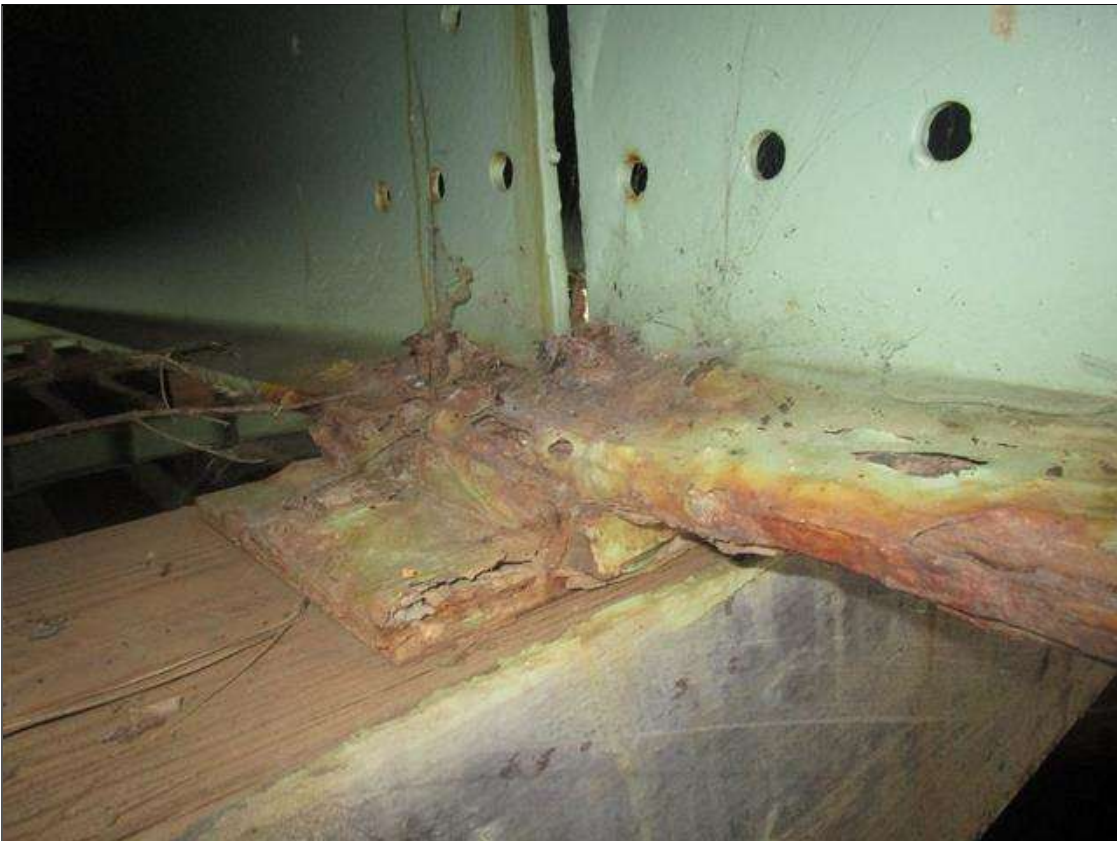
Span 5 Beam 5 - Near Bearing: ANCHOR BOLT COMPLETELY CORRODED, PAR
