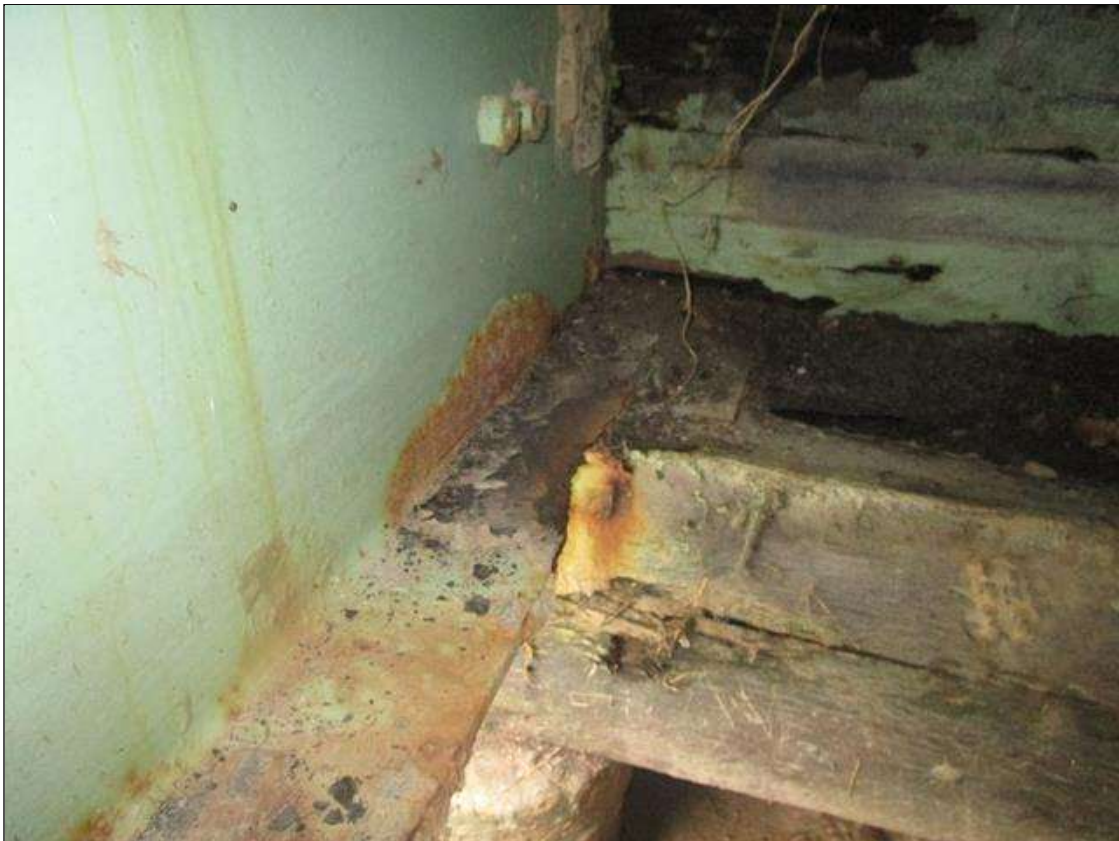
Span 5 Beam 1: SPAN 6 AT END BENT 2, 3FT X 1IN WIDE AREA OF 100% SECTION LOSS IN BOTTOM FLANGE, PAR
