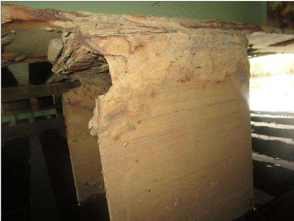
Bent 3 Pile 3: 2IN LONG X 1IN WIDE X 100% SECTION LOSS OF BOTH EDGES AT BOTH FLANGES AT TOP OF PILE. 1/8IN SECTION LOSS IN TOP PLATE, PAR
