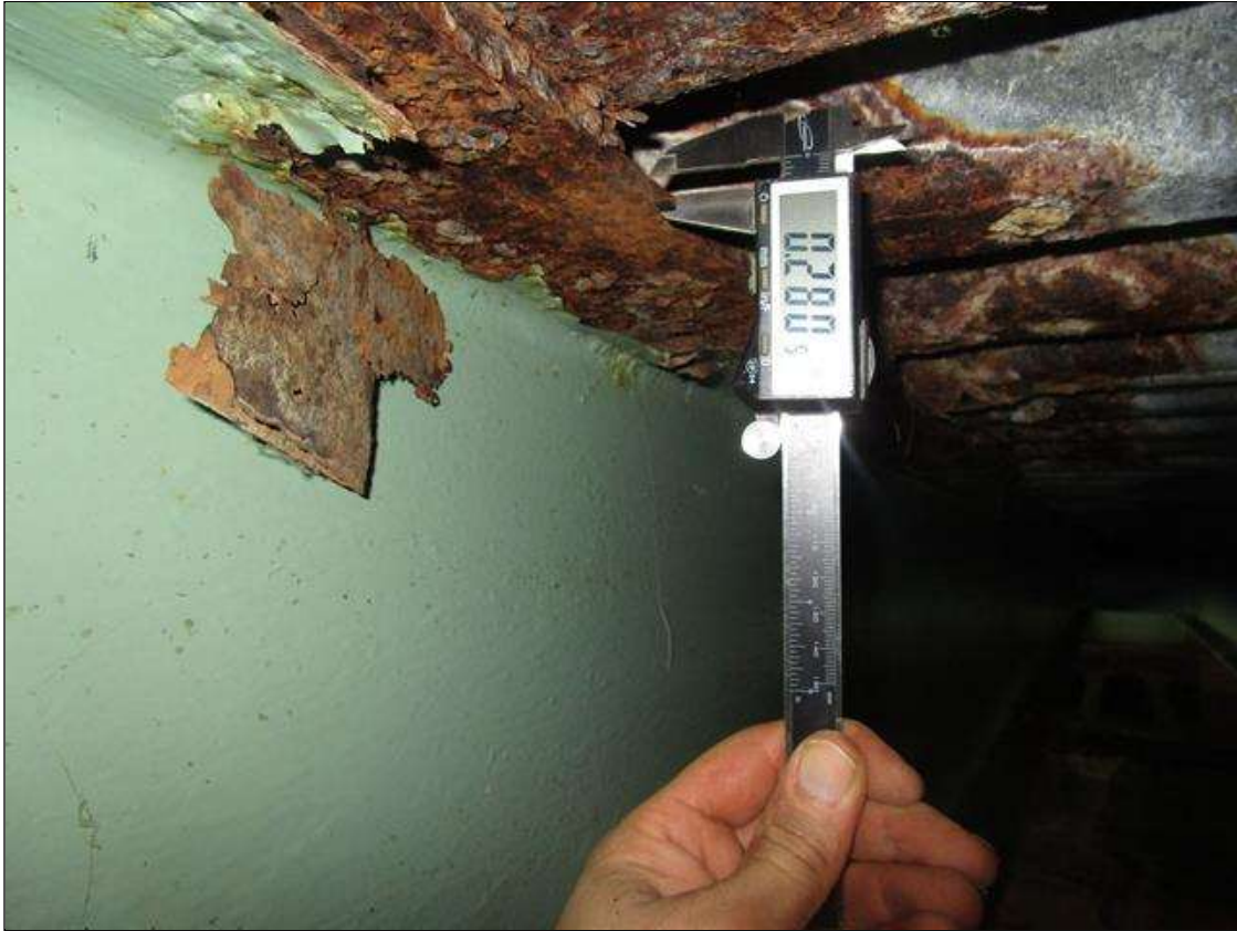
Span 5 Beam 9: SPAN 5, 12FT AT MIDSPAN, SECTION LOSS IN TOP AND BOTTOM FLANGES DOWN TO 0.280IN REMAINING, PAR
