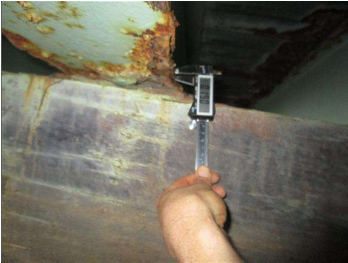
Span 3 Beam 2: SPAN 4, AT BENT 4, 1FT AREA OF SECTION LOSS DOWN TO 0.19IN REMAINING IN BOTTOM FLANGE, PAR
