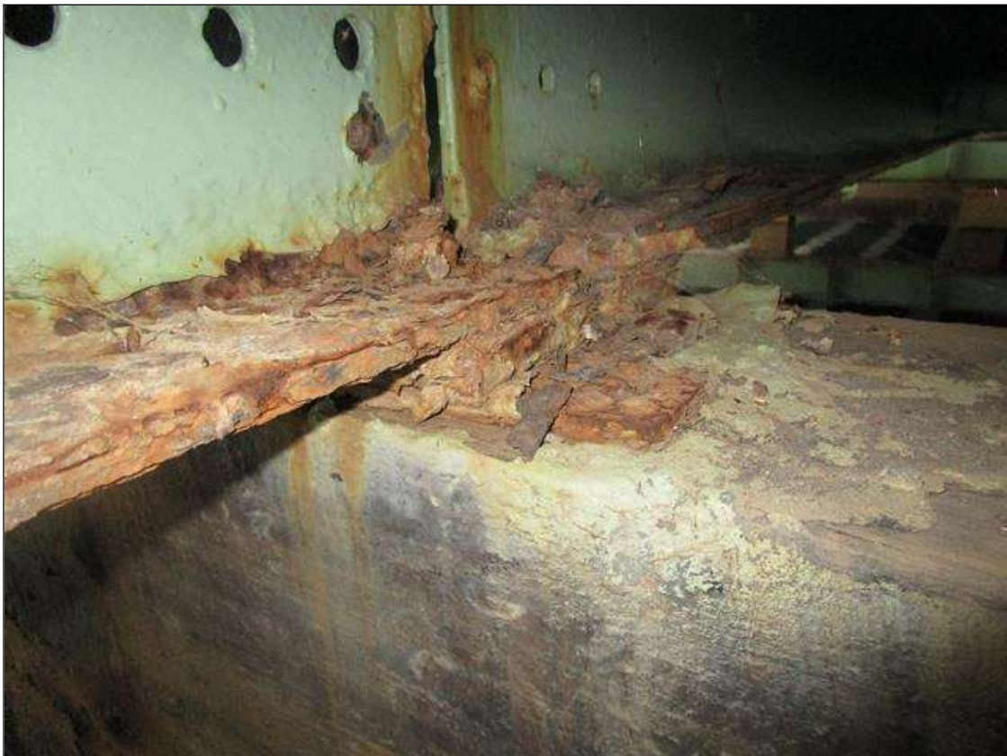
Span 5 Beam 8 - Near Bearing: 1/8IN SECTION LOSS, 3/8IN REMAINING, PAR
