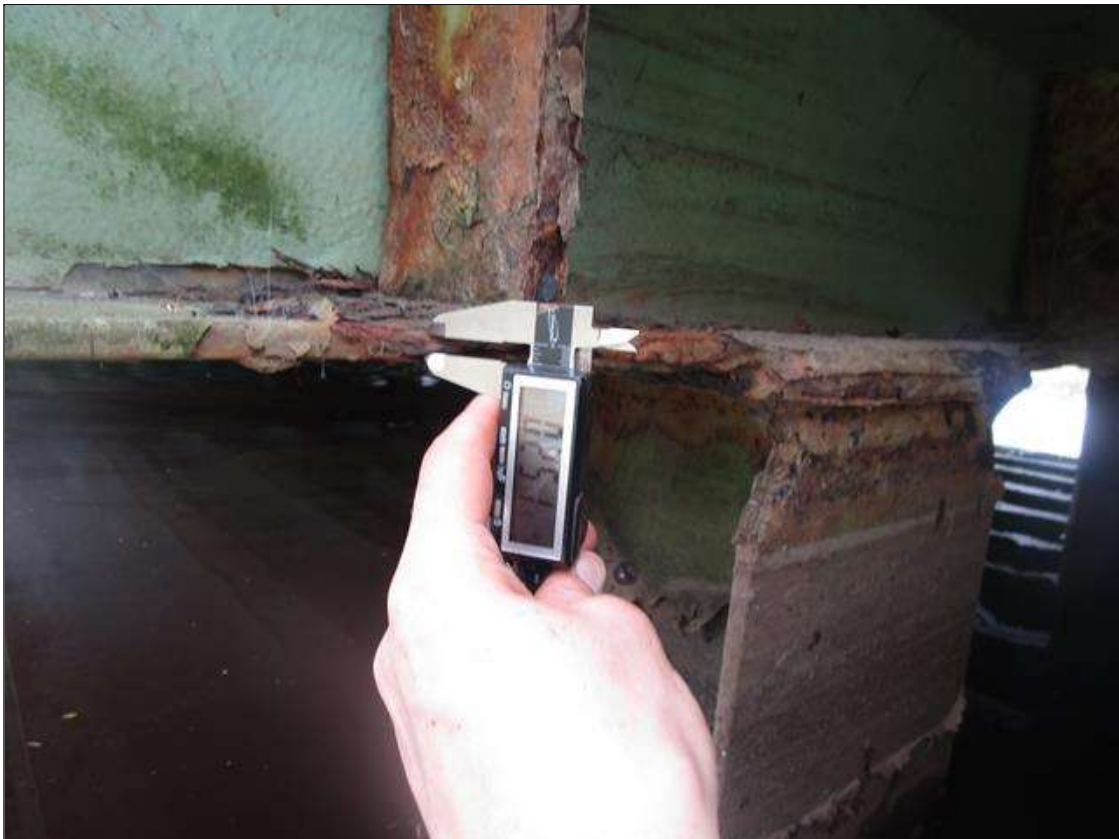
Bent 1 Cap 1: 3FT OF CORROSION IN BOTTOM FLANGE AT BEAM 1, BEAM 2 AND PILE 1. 0.251IN REMAINING, PAR
