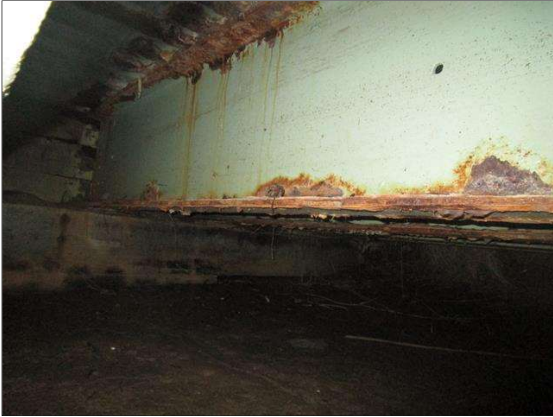
Span 5 Beam 9: SPAN 6, INTERMITTENT FULL LENGTH AREA OF SECTION LOSS IN BOTTOM FLANGE DOWN TO 5/16IN REMAINING, PAR
