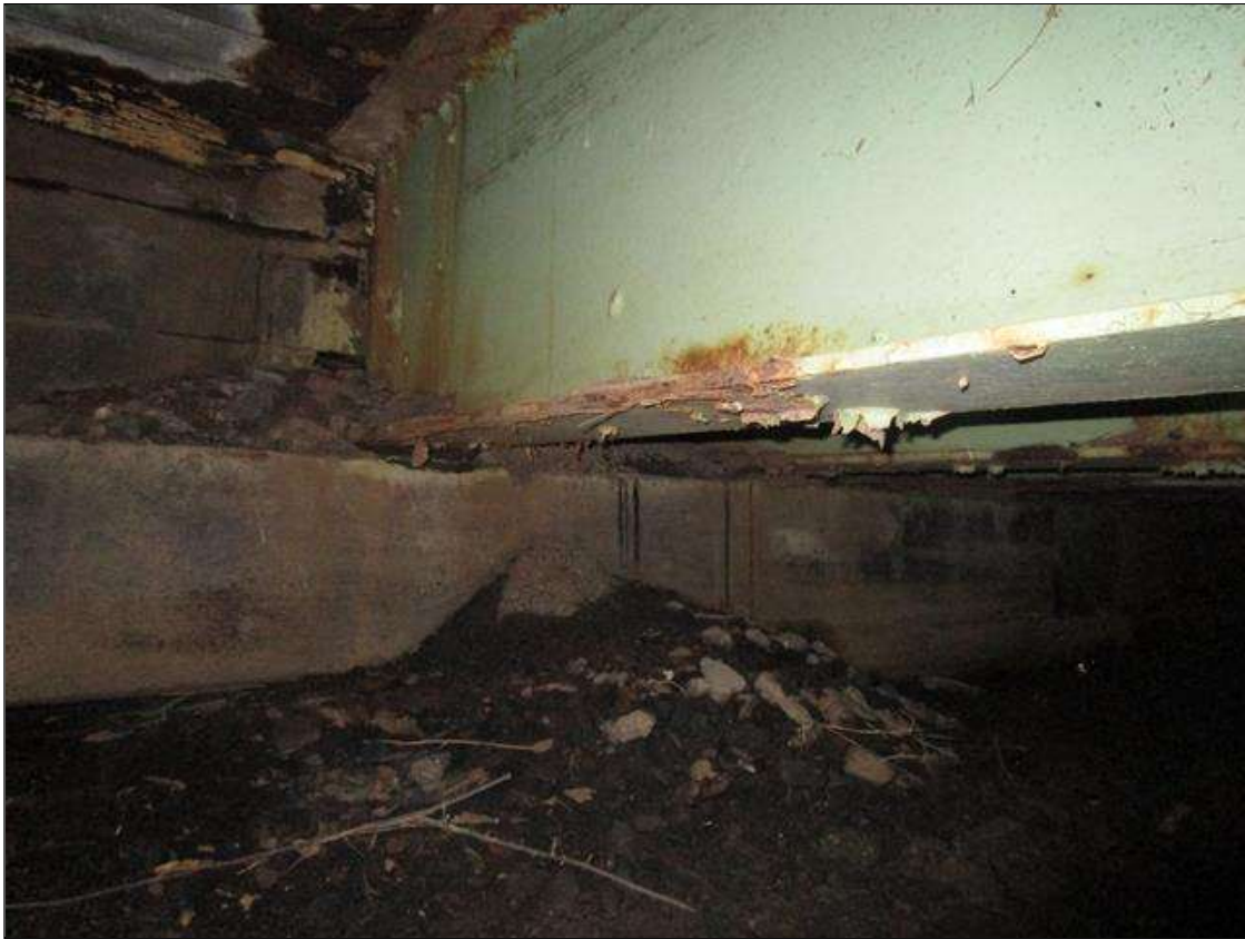
Span 5 Beam 6: SPAN 6, AT END BENT 2, 3FT AREA OF SECTION LOSS DOWN TO 5/16IN REMAINING IN BOTTOM FLANGE, PAR
