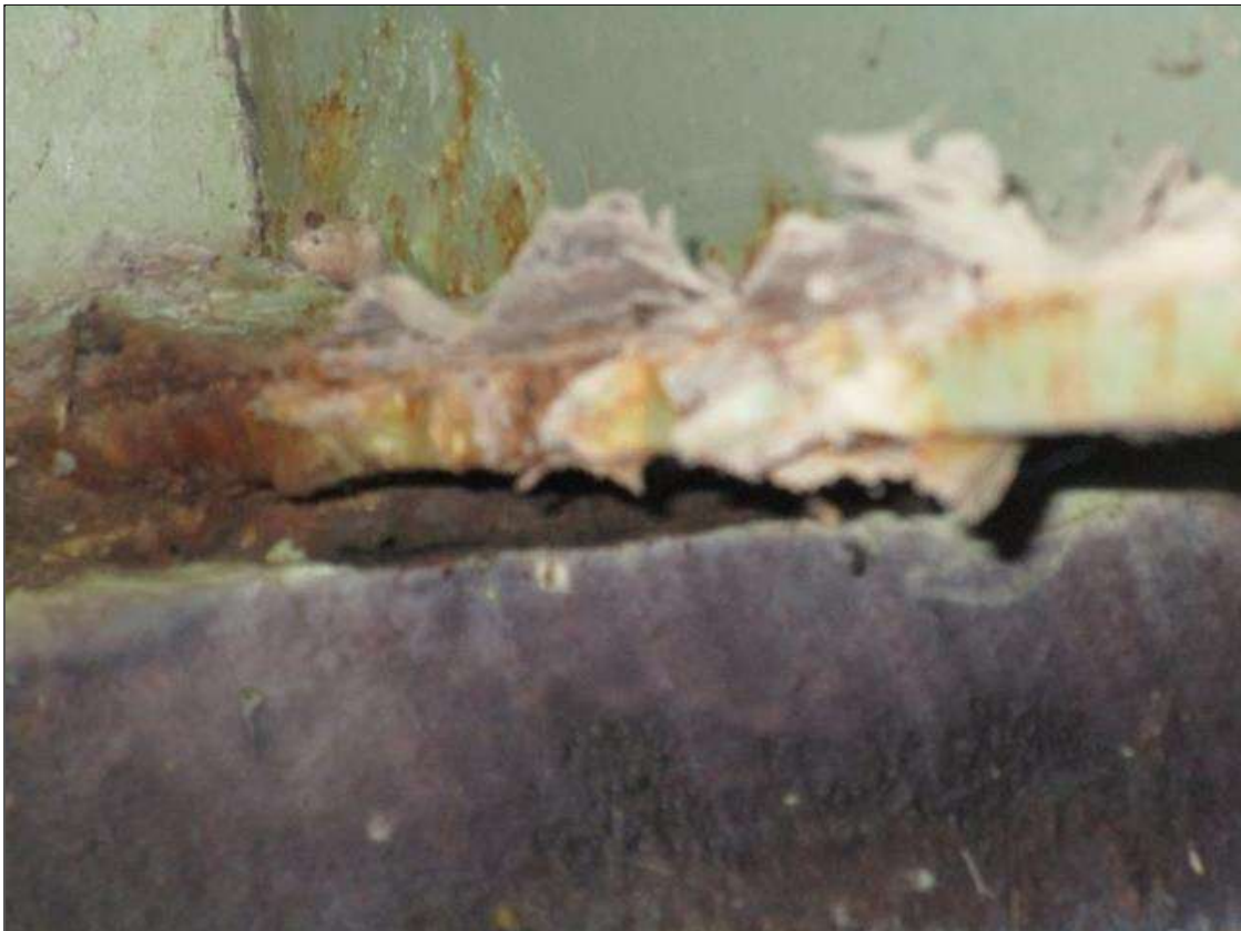
Span 1 Beam 11: SPAN 1, AT END BENT 1, 2FT AREA OF SECTION LOSS IN BOTTOM FLANGE DOWN TO 3/16IN REMAINING, PAR
