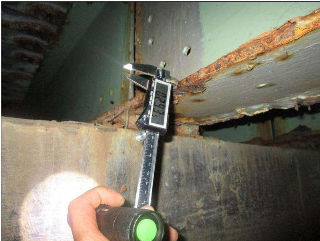
Span 1 Beam 7: SPAN 2, INTERMITTENT FULL LENGTH, SECTION LOSS IN BOTTOM FLANGE DOWN TO 0.293IN REMAINING, PAR
