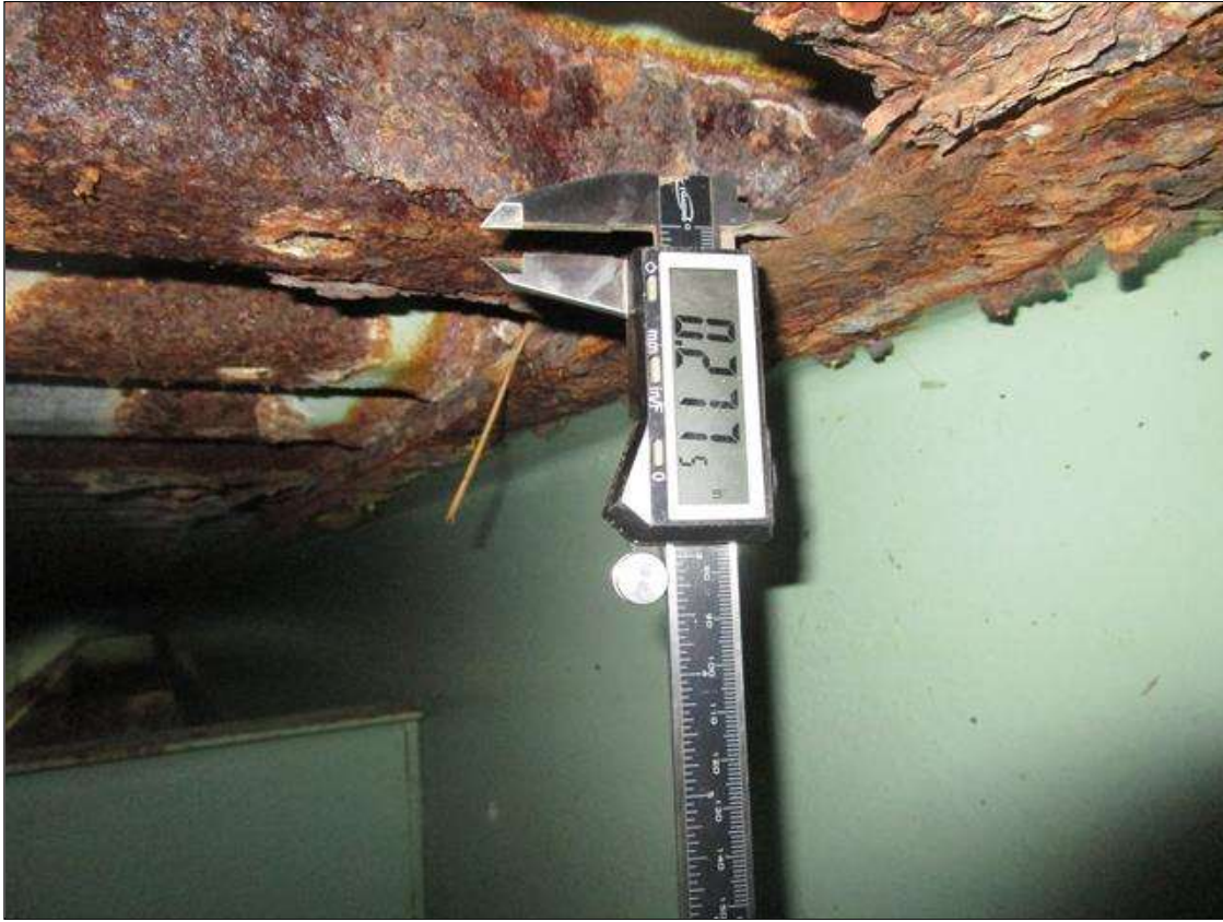
Span 3 Beam 9: SPAN 4, AT BENT 4, 7FT AREA OF SECTION LOSS DOWN TO 0.277IN REMAINING IN TOP FLANGE, PAR
