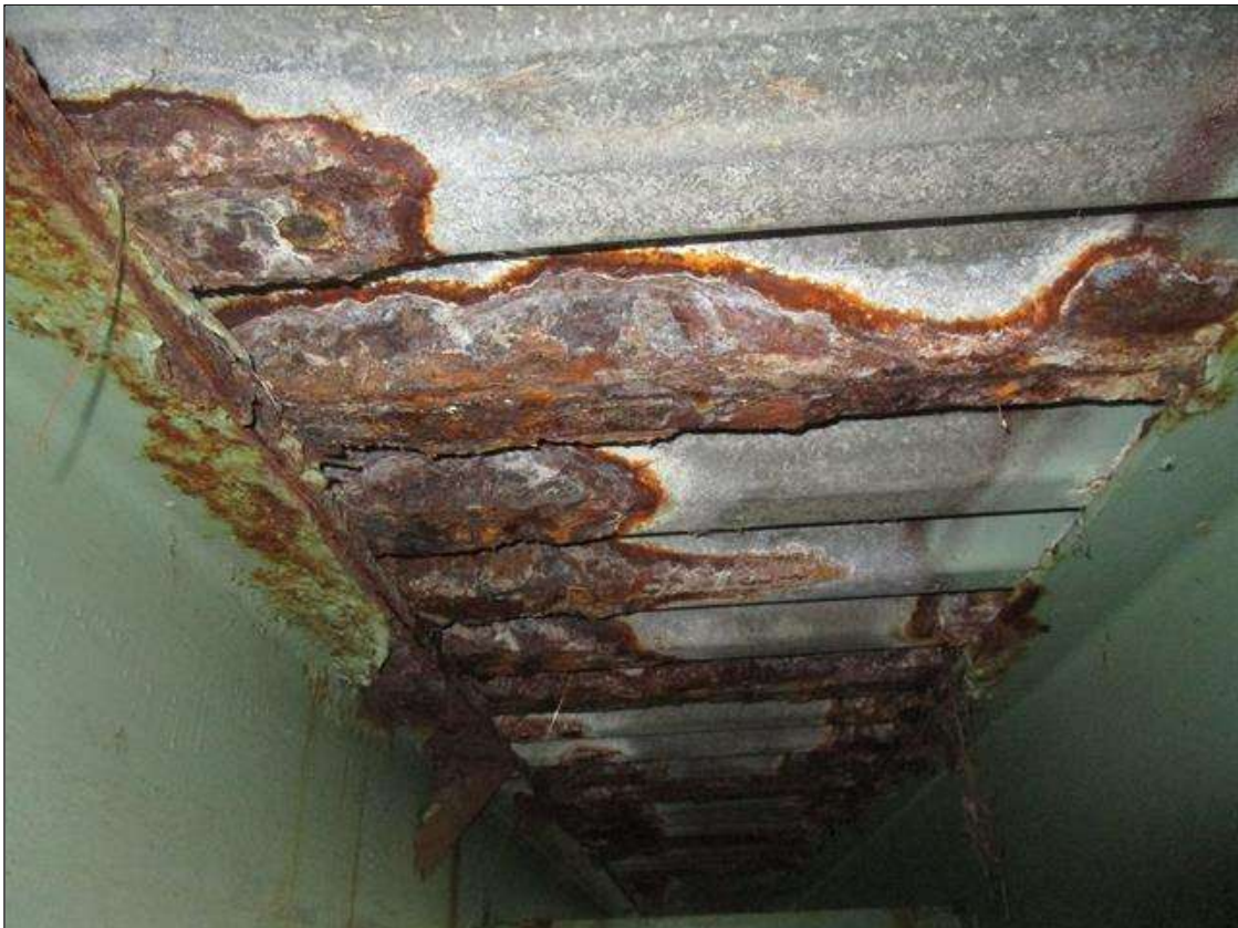
Span 6 Deck: UNDERSIDE OF PLANK DECK, BAYS 3-4, 20SF OF DELAMINATED STEEL WITH 25% SECTION LOSS, PAR
