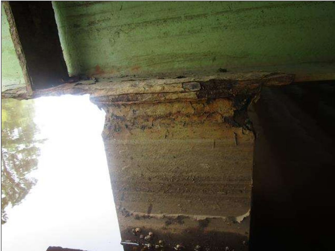
Bent 1 Pile 1: 2IN LONG X 1IN WIDE X 100% SECTION LOSS OF BOTH EDGES AT BOTH FLANGES AT TOP OF PILE. 1/8IN SECTION LOSS IN TOP PLATE, PAR
