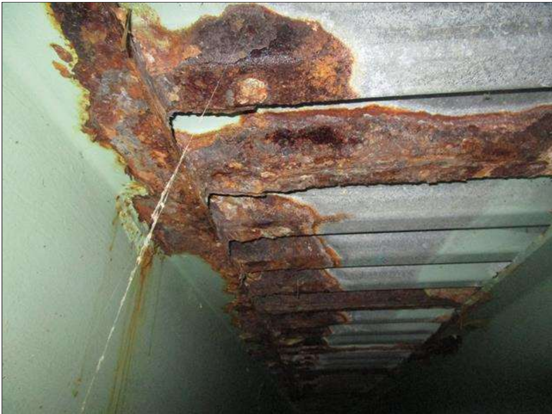
Span 4 Deck: BAY 8, 7FT X 1FT AREA OF 25% SECTION LOSS, PAR
