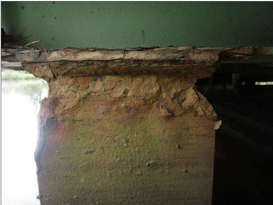
Bent 3 Pile 1: 2IN LONG X 1IN WIDE X 100% SECTION LOSS OF BOTH EDGES AT BOTH FLANGES AT TOP OF PILE. 1/8IN SECTION LOSS IN TOP PLATE, PAR
