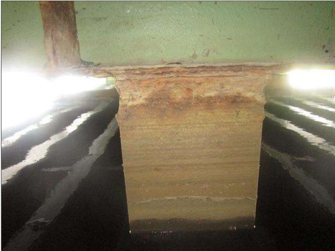
Bent 1 Pile 3: 2IN LONG X 1IN WIDE X 100% SECTION LOSS OF BOTH EDGES AT BOTH FLANGES AT TOP OF PILE. 1/8IN SECTION LOSS IN TOP PLATE, PAR
