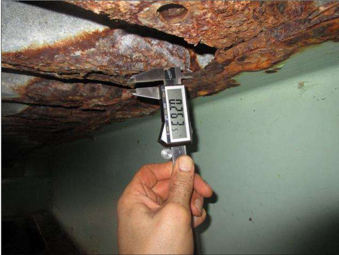
Span 3 Beam 3: SPAN 3, INTERMITTENT FULL LENGTH CORROSION WITH SECTION LOSS DOWN TO 0.263IN REMAINING IN THE TOP FLANGE, PAR
