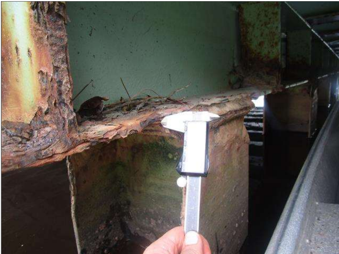
Bent 3 Cap 1: AT PILE 1, 1/2IN WIDE X 100% SECTION LOSS AT BOTTOM FLANGE, PAR
