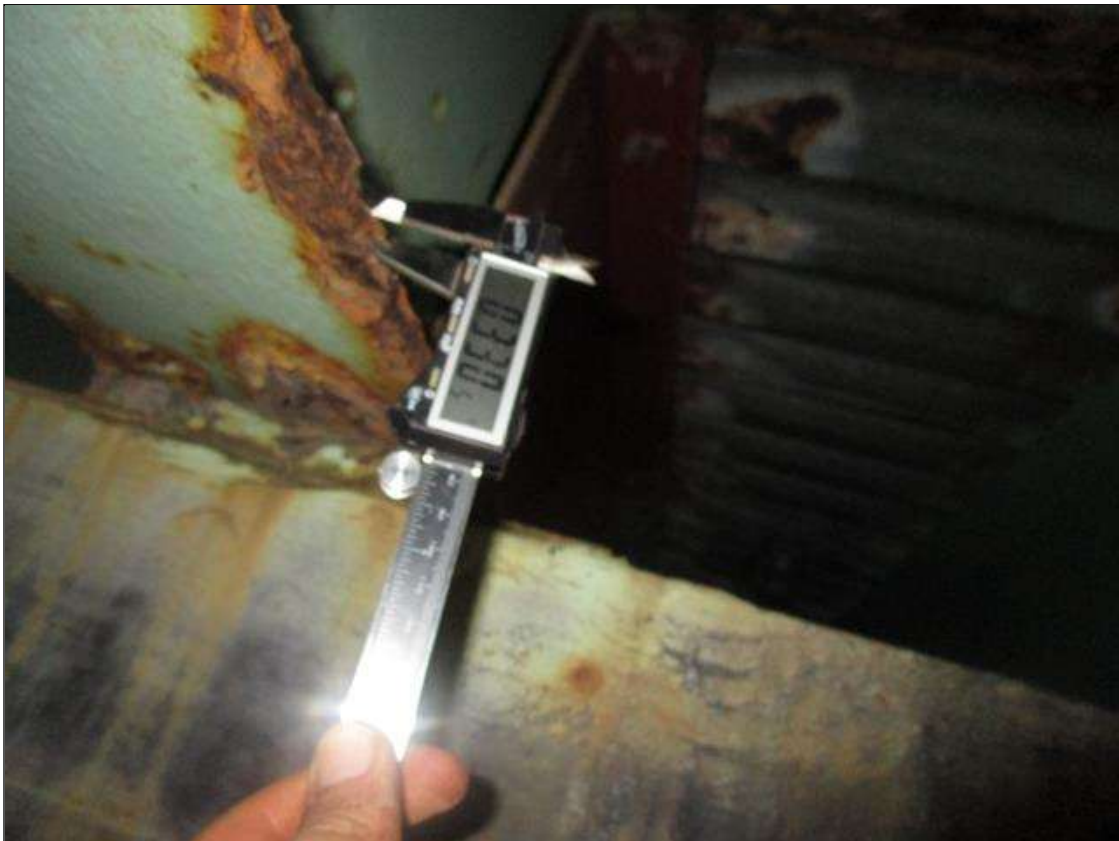
Span 3 Beam 4: SPAN 3, AT BENT 2, 4FT AREA OF SECTION LOSS DOWN TO 0.33IN REMAINING IN THE BOTTOM FLANGE, PAR
