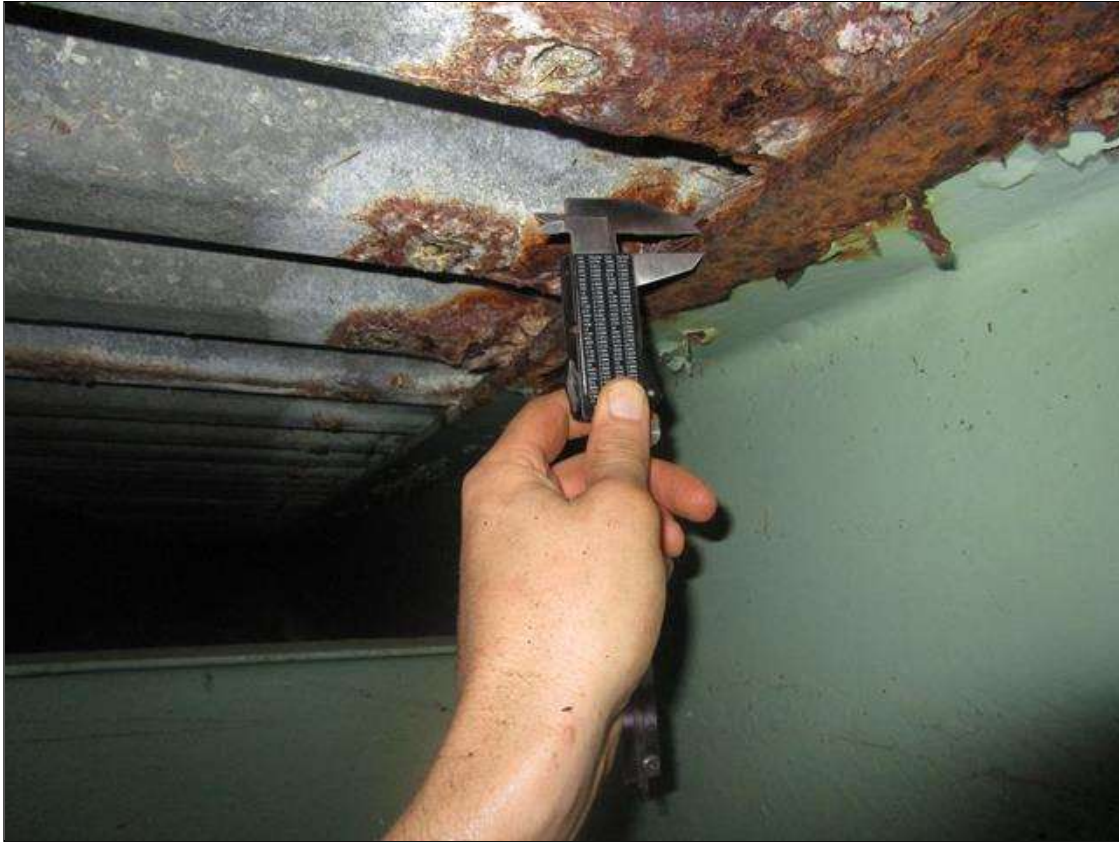
Span 5 Beam 7: SPAN 6, 3FT FROM BENT 5, 3FT LONG AREA OF SECTION LOSS DOWN TO 0.33IN REMAINING IN TOP FLANGE, PAR
