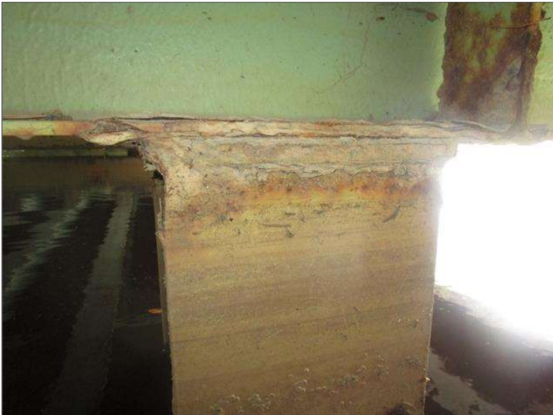
Bent 1 Pile 5: 2IN LONG X 1IN WIDE X 100% SECTION LOSS OF BOTH EDGES AT BOTH FLANGES AT TOP OF PILE. 1/8IN SECTION LOSS IN TOP PLATE, PAR
