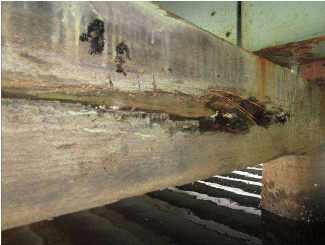
Bent 2 Cap 2: WEST FACE OF CAP BELOW BAYS 1 AND 2, 3FT LONG X 6IN HIGH X 2IN DEEP DECAYED AREA, PAR
