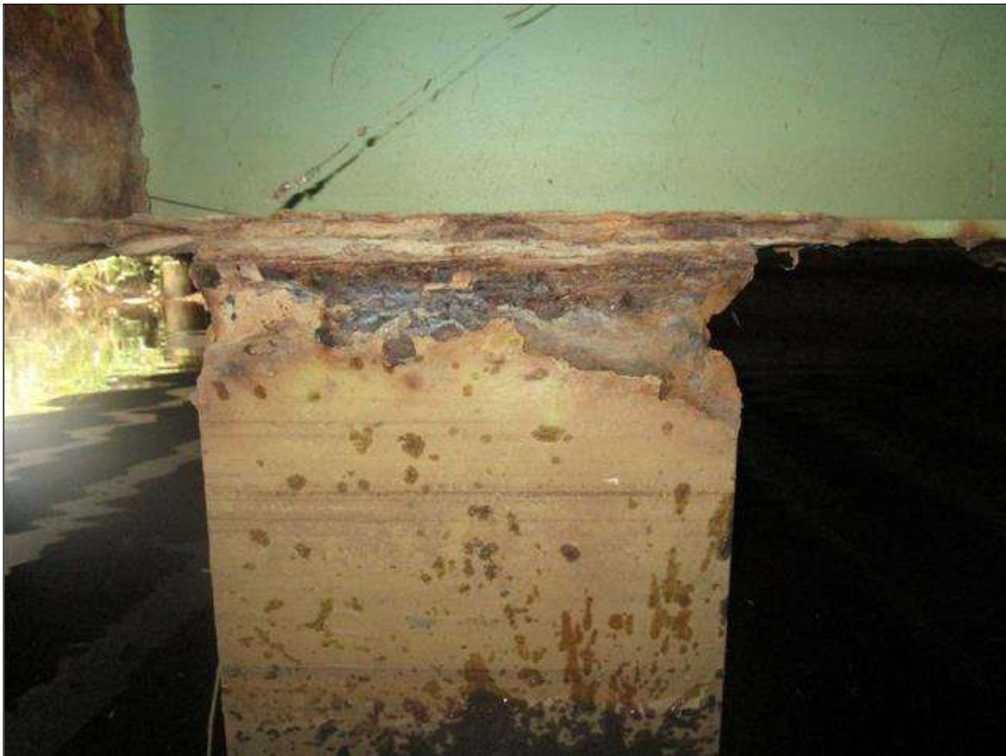
Bent 5 Pile 3: 2IN LONG X 1IN WIDE X 100% SECTION LOSS OF BOTH EDGES AT BOTH FLANGES AT TOP OF PILE. 1/8IN SECTION LOSS IN TOP PLATE, PAR
