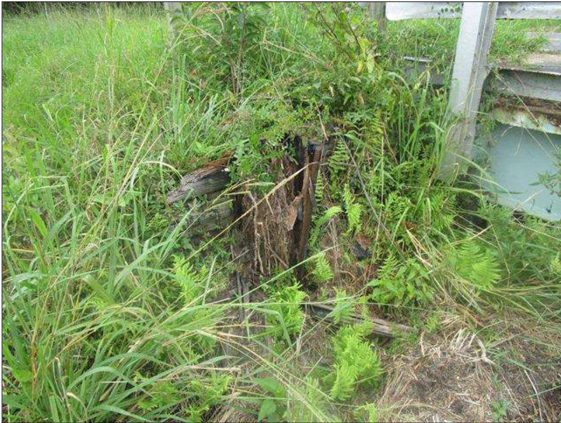
END BENT 1 ABUTMENT: END BENT 1 RIGHT SIDE, 100% DECAY IN ABUTMENT PILE, PAR
