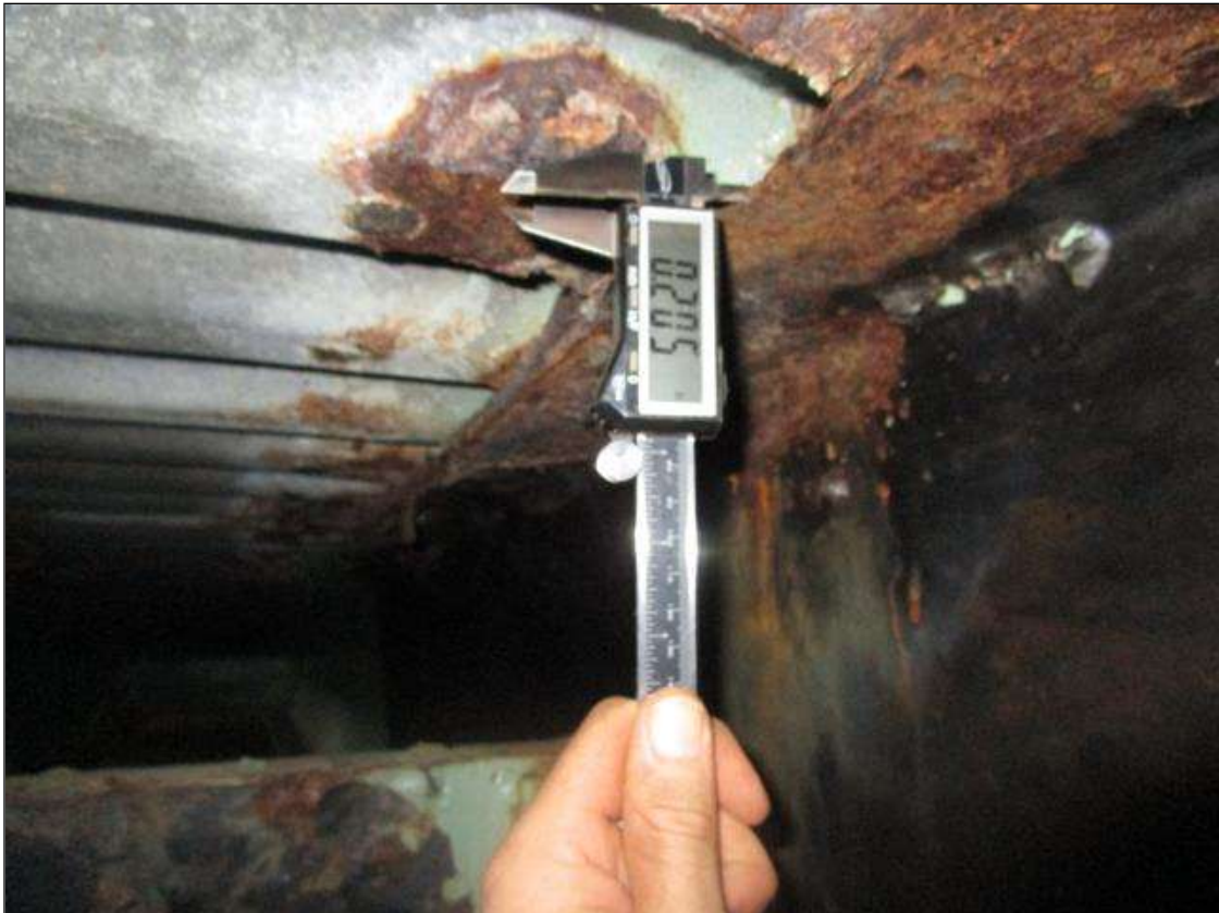
Span 5 Beam 6: SPAN 5, INTERMITTENT FULL LENGTH CORROSION WITH SECTION LOSS DOWN TO 0.205IN REMAINING IN TOP FLANGE, PAR
