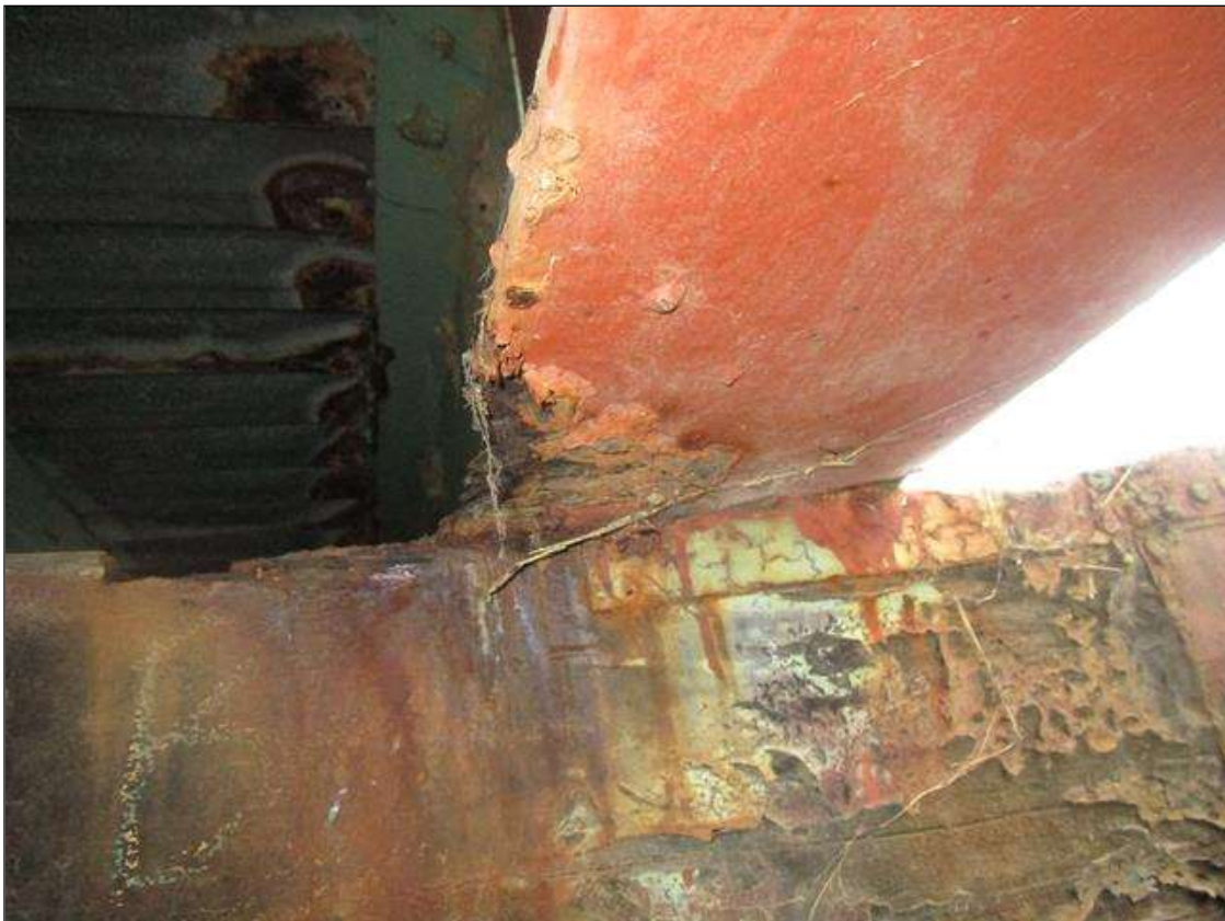
Span 1 Beam 12: SPAN 2, AT BENT 2, 1FT X 1IN WIDE AREA OF 100% SECTION LOSS IN BOTTOM FLANGE, PAR
