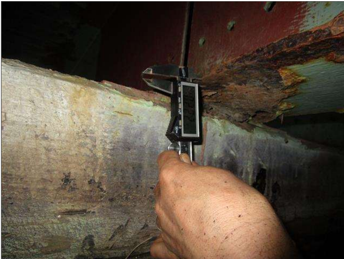
Span 1 Beam 2: SPAN 2, AT BENT 2, 1FT AREA OF SECTION LOSS DOWN 0.222IN REMAINING IN BOTTOM FLANGE, PAR
