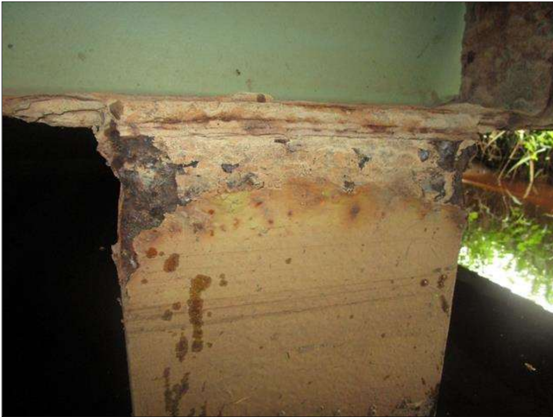
Bent 5 Pile 5: 2IN LONG X 1IN WIDE X 100% SECTION LOSS OF BOTH EDGES AT BOTH FLANGES AT TOP OF PILE. 1/8IN SECTION LOSS IN TOP PLATE, PAR
