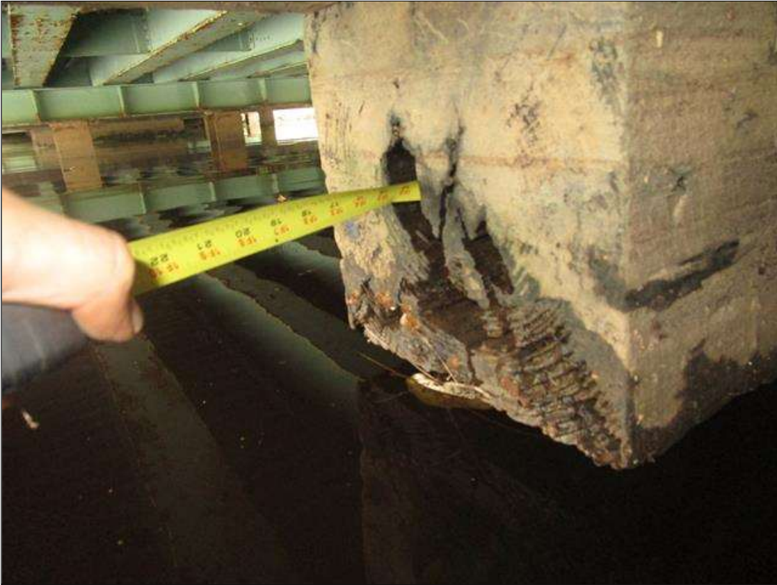
Bent 4 Cap 2: SOUTH END OF THE SUB CAP, 10IN HIGH X 12IN WIDE X 14IN DEEP DECAY IN PILE 4, PAR
