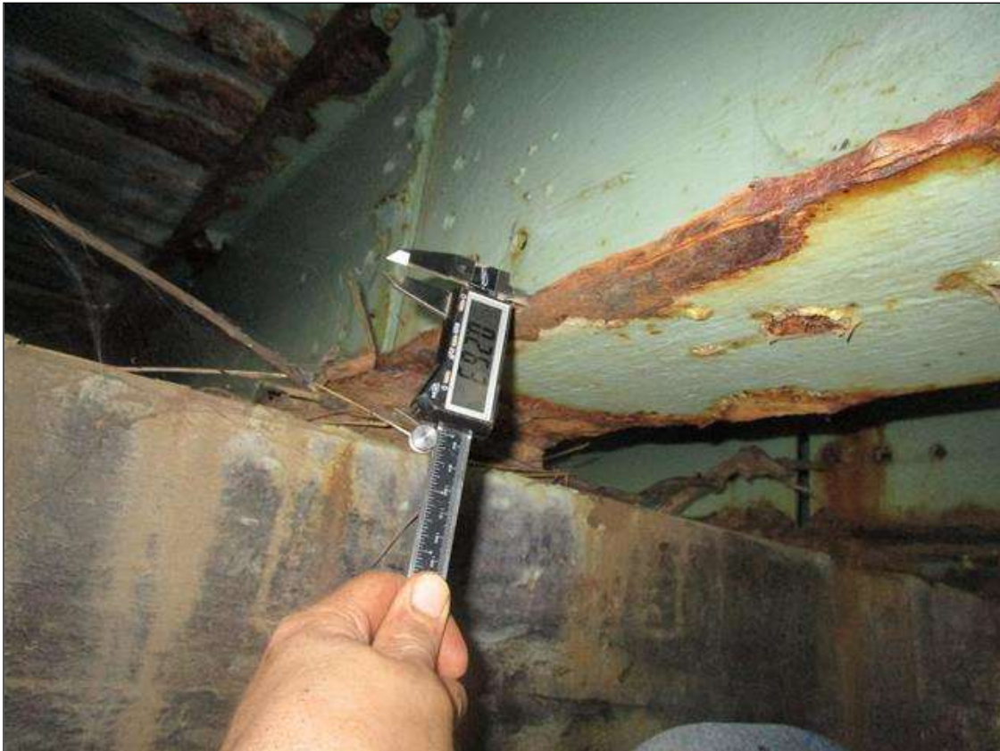
Span 3 Beam 6: SPAN 4, AT BENT 4, 2FT AREA OF SECTION LOSS DOWN TO 0.263IN REMAINING IN BOTTOM FLANGE, PAR
