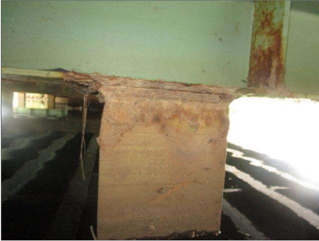
Bent 3 Pile 4: 2IN LONG X 1IN WIDE X 100% SECTION LOSS OF BOTH EDGES AT BOTH FLANGES AT TOP OF PILE. 1/8IN SECTION LOSS IN TOP PLATE, PAR
