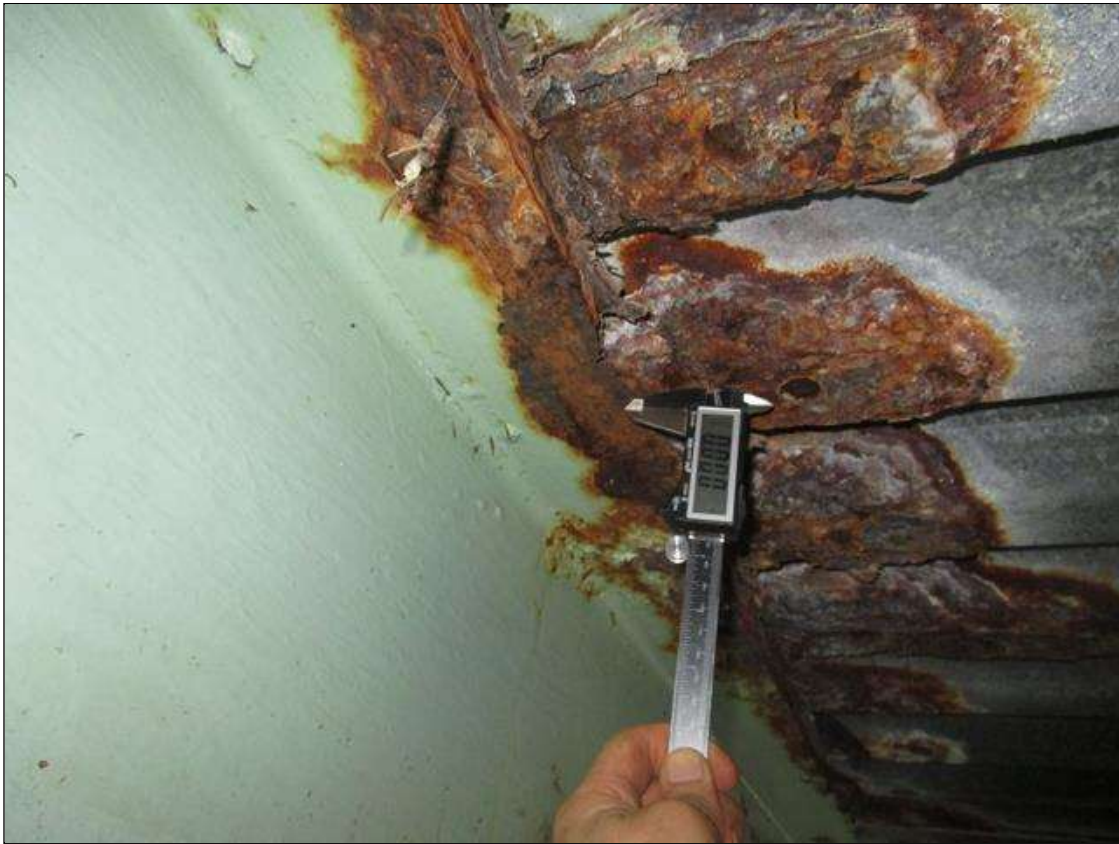
Span 5 Beam 3: SPAN 6, INTERMITTENT FULL LENGTH X 1/2IN WIDE AREA OF CORROSION WITH 100% SECTION LOSS IN BOTTOM AND TOP FLANGE, PAR
