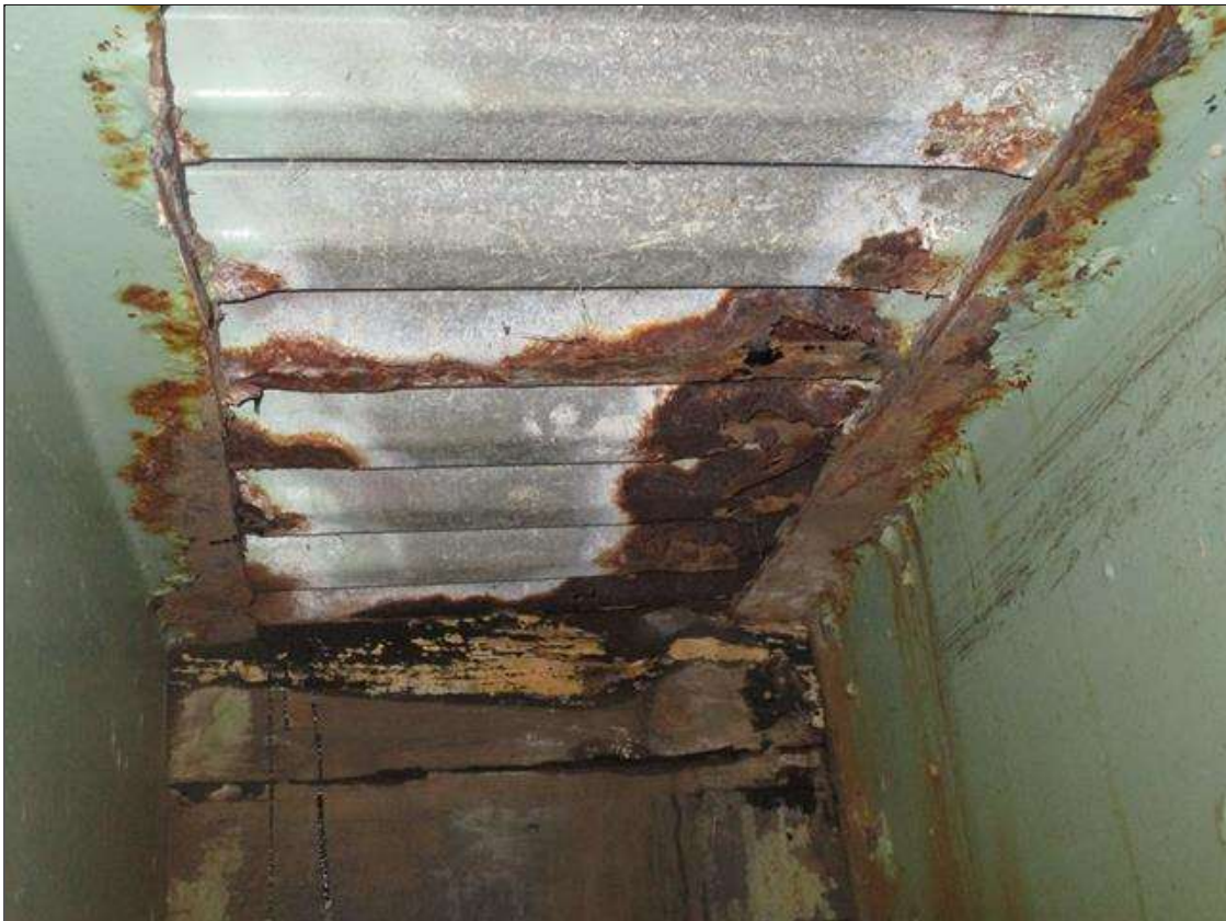
Span 6 Deck: BAY 5, AT END BENT 2, 2FT X 1FT AREA OF 100% SECTION LOSS, PAR
