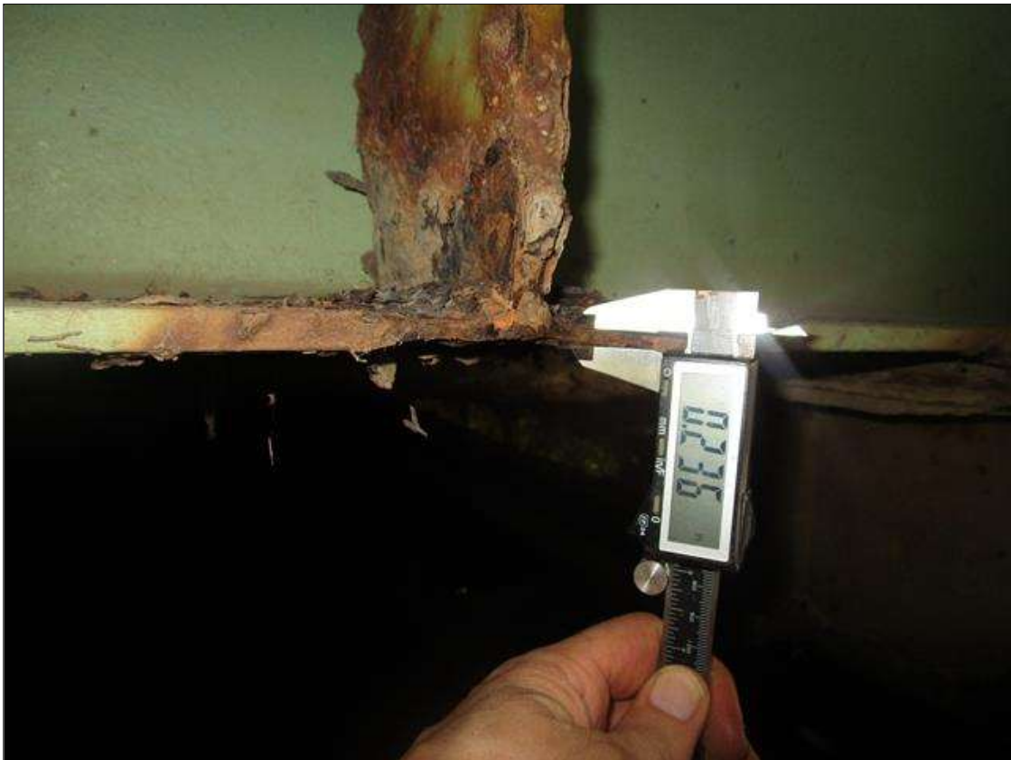
Bent 5 Cap 1: AT BEAM 9, SECTION LOSS IN BOTTOM FLANGE DOWN TO 0.236IN REMAINING, PAR
