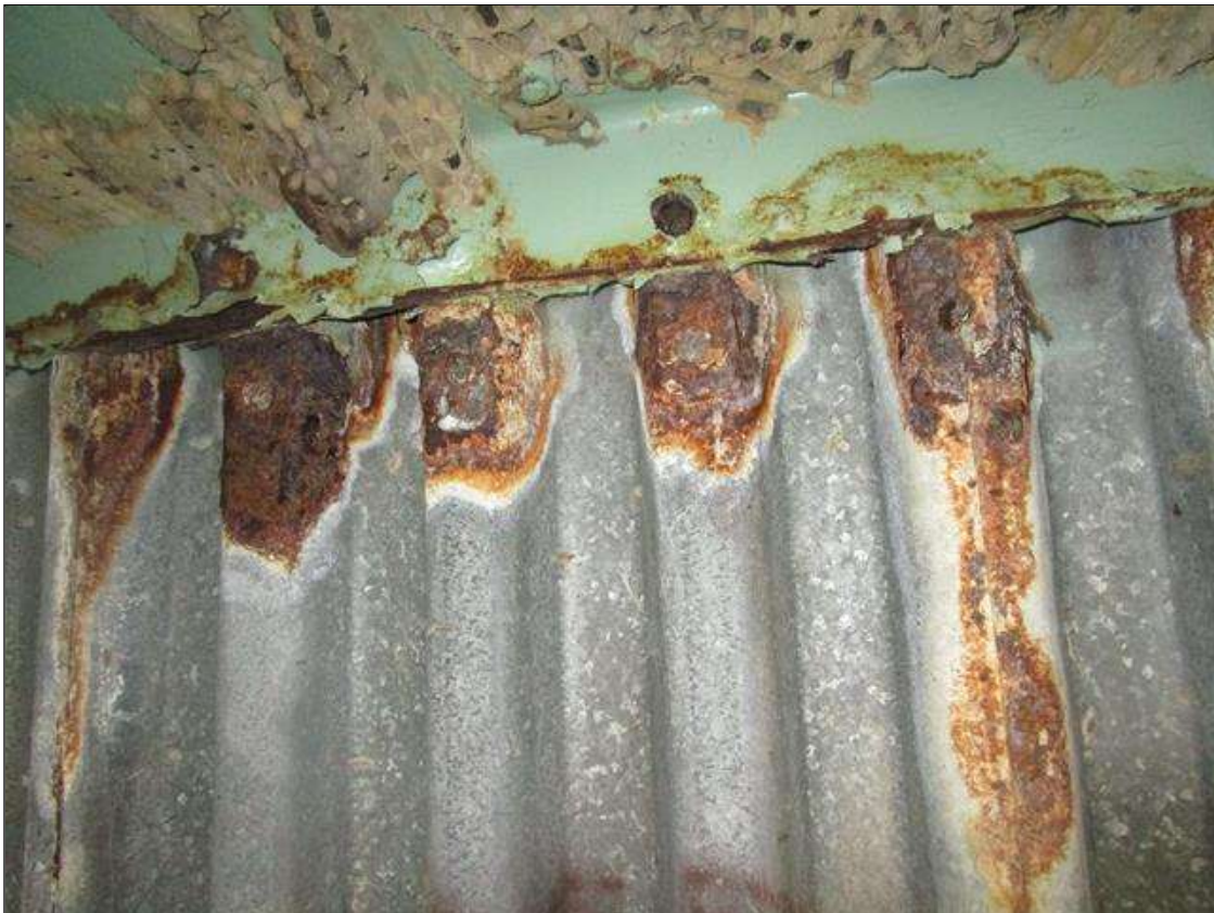
Span 6 Deck: BAY 11, 2FT X 1FT AREA OF 50% SECTION LOSS, PAR
