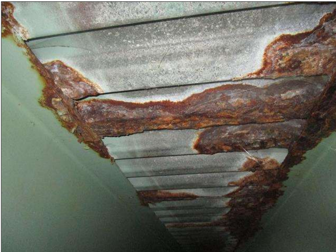
Span 3 Deck: BAYS 2-3, 10FT X 2FT AREA OF 25% SECTION LOSS, PAR
