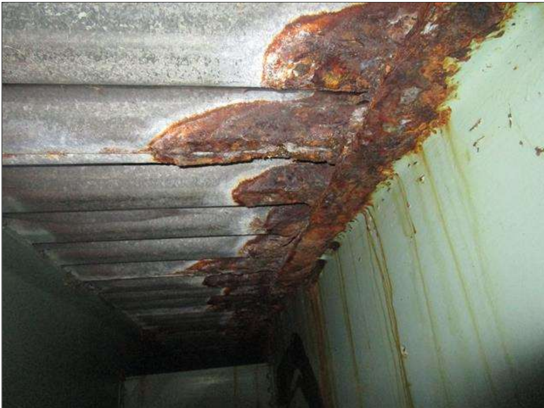
Span 1 Deck: BAYS 3-4, 20SF OF 50% SECTION LOSS, PAR
