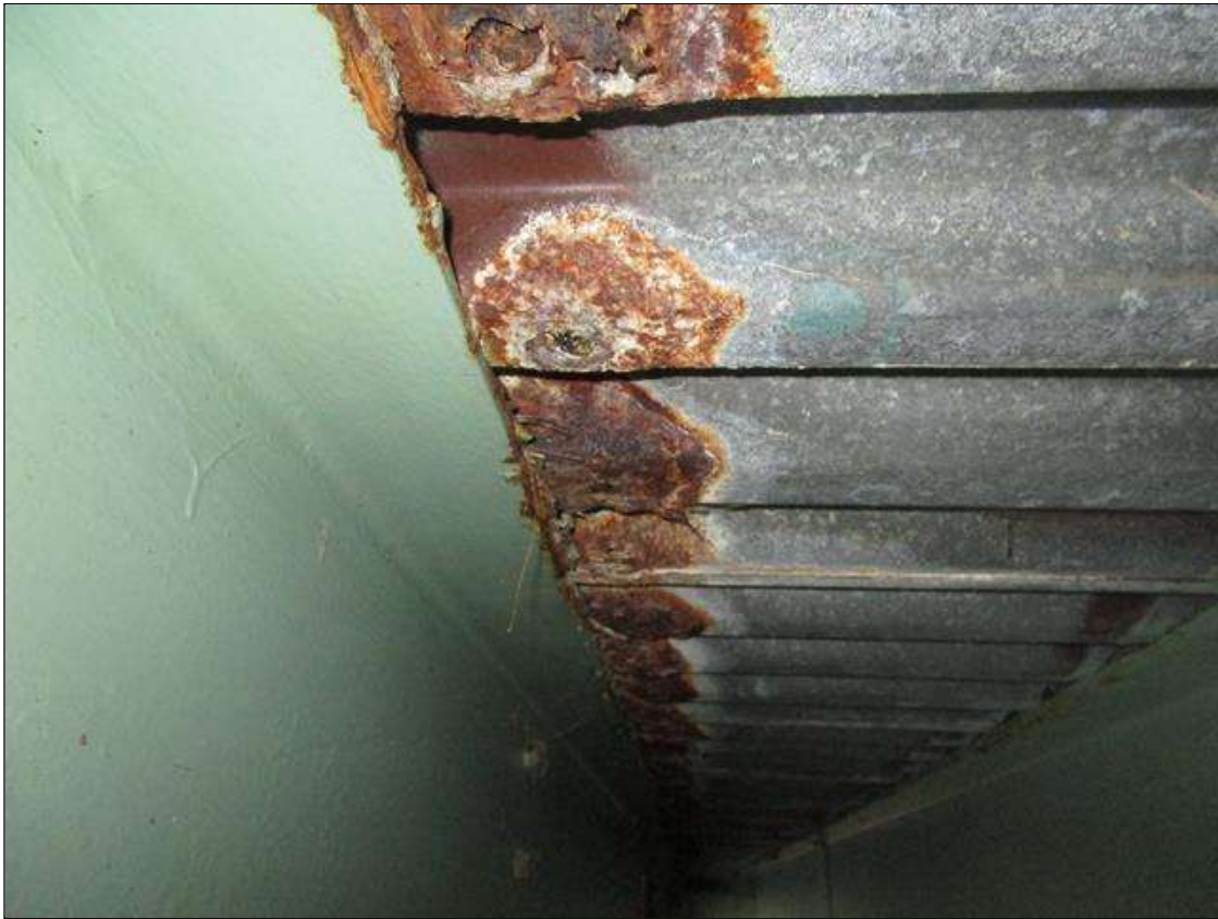
Span 3 Deck: BAY 11, 20FT X 6IN, CORROSION WITH 25% SECTION LOSS, PAR
