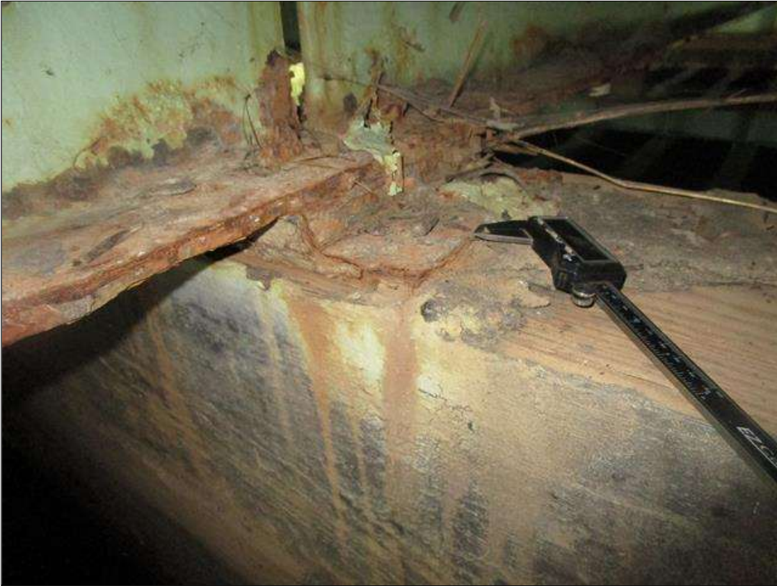
Span 5 Beam 6 - Near Bearing: FULL LENGTH X FULL WIDTH AREA OF DELAMINATED STEEL WITH 1/8IN SECTION LOSS. DOWN TO 3/8IN REMAINING, PAR
