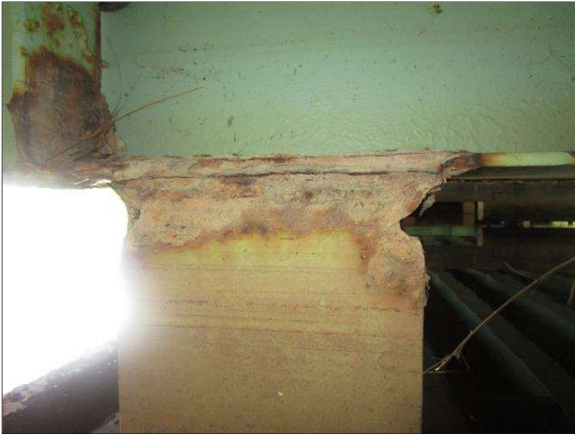
Bent 3 Pile 2: 2IN LONG X 1IN WIDE X 100% SECTION LOSS OF BOTH EDGES AT BOTH FLANGES AT TOP OF PILE. 1/8IN SECTION LOSS IN TOP PLATE, PAR
