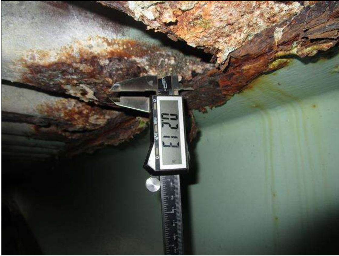
Span 3 Beam 4: SPAN 4, MIDSPAN, 3FT OF CORROSION WITH SECTION LOSS IN TOP FLANGE DOWN TO 0.213IN REMAINING, PAR
