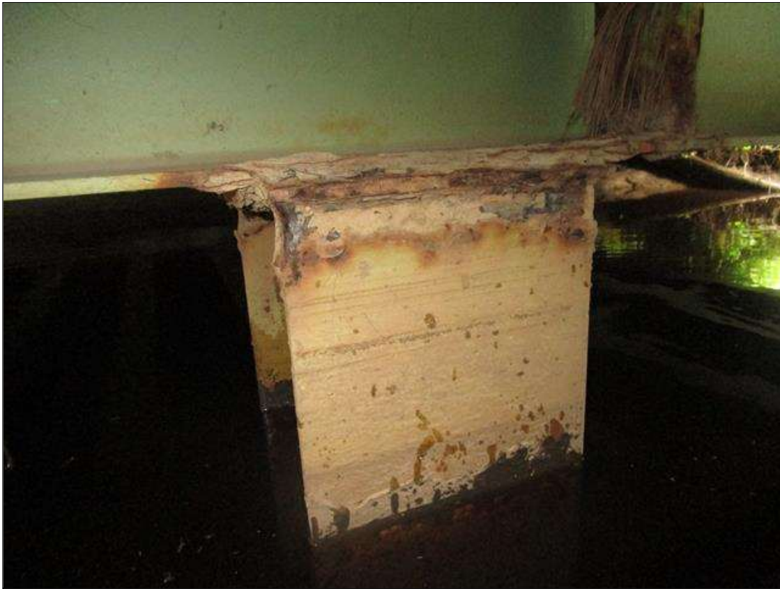
Bent 5 Pile 4: 2IN LONG X 1IN WIDE X 100% SECTION LOSS OF BOTH EDGES AT BOTH FLANGES AT TOP OF PILE. 1/8IN SECTION LOSS IN TOP PLATE, PAR
