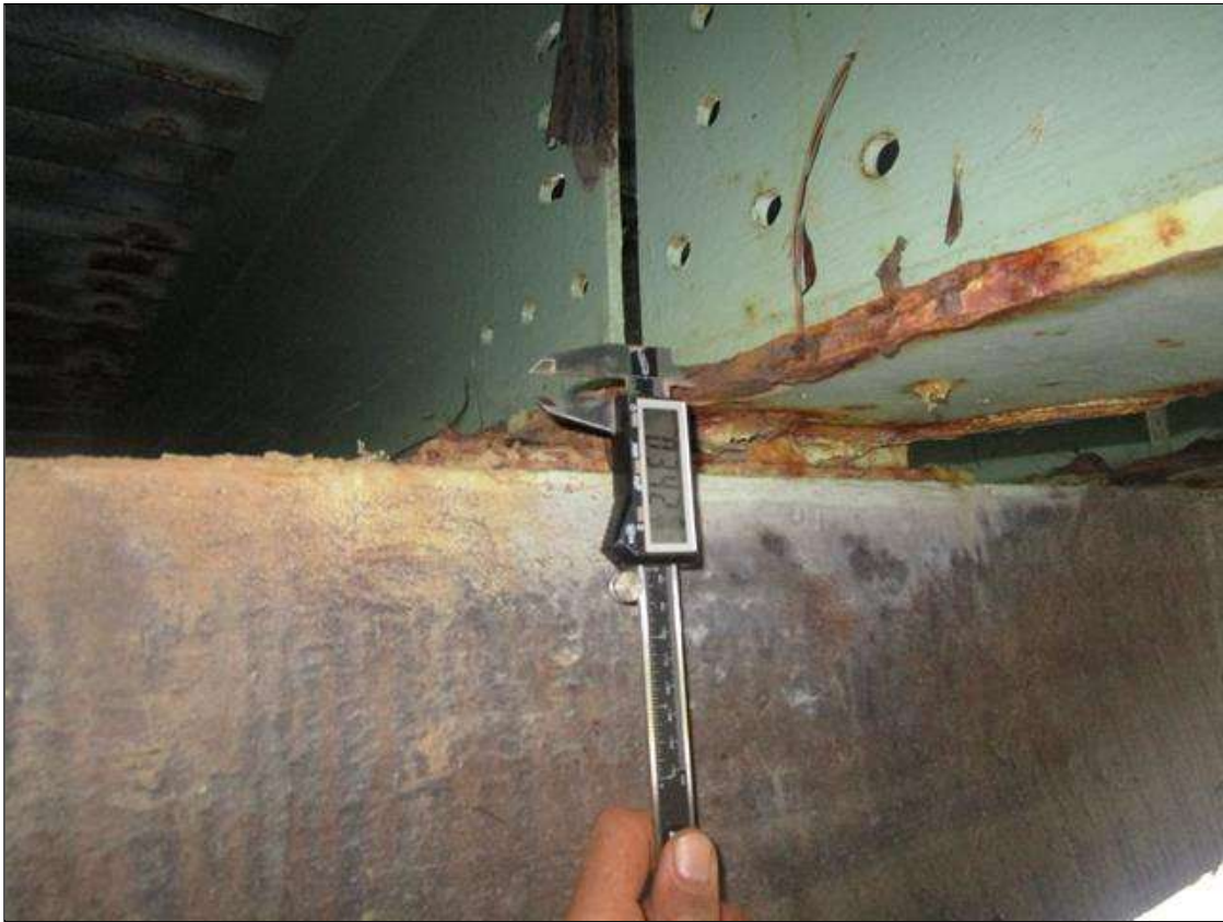
Span 3 Beam 10: SPAN 4, 2FT OF SECTION LOSS DOWN TO 0.342IN REMAINING IN TOP AND BOTTOM FLANGE, PAR
