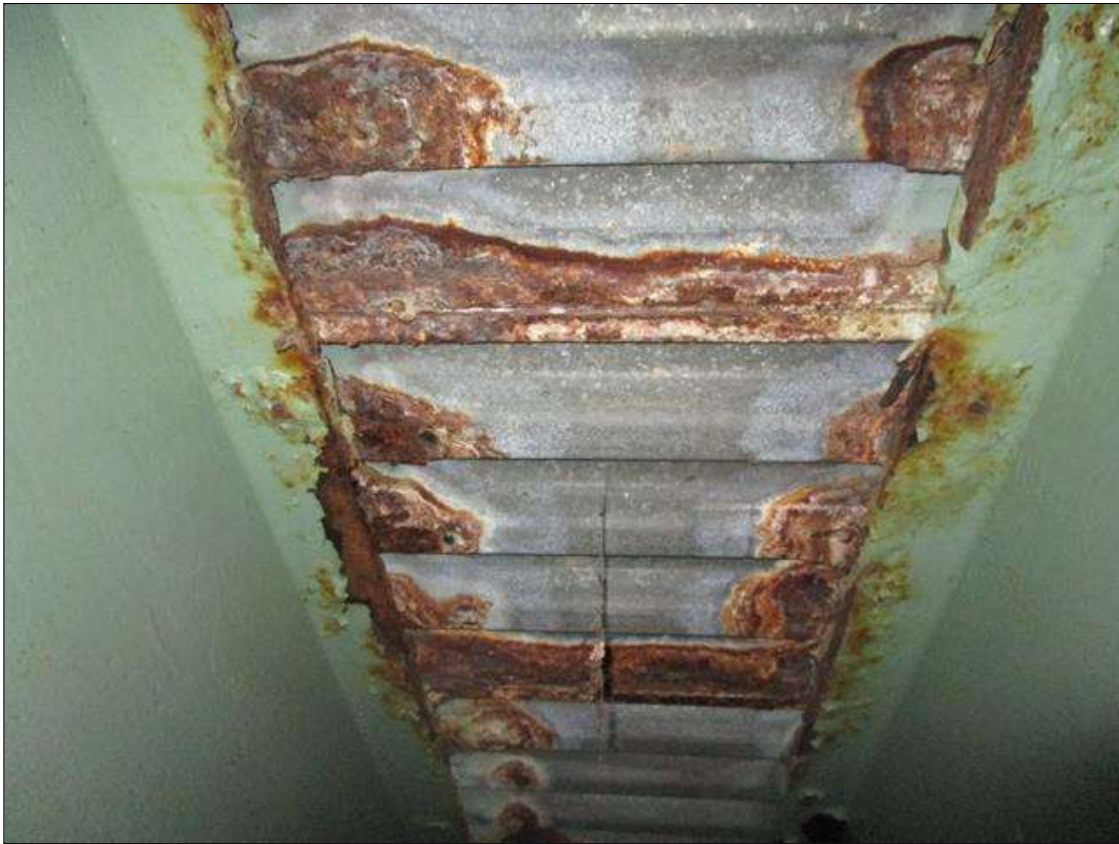
Span 6 Deck: BAY 7, 4FT X 2FT AREA OF 45% SECTION LOSS, PAR
