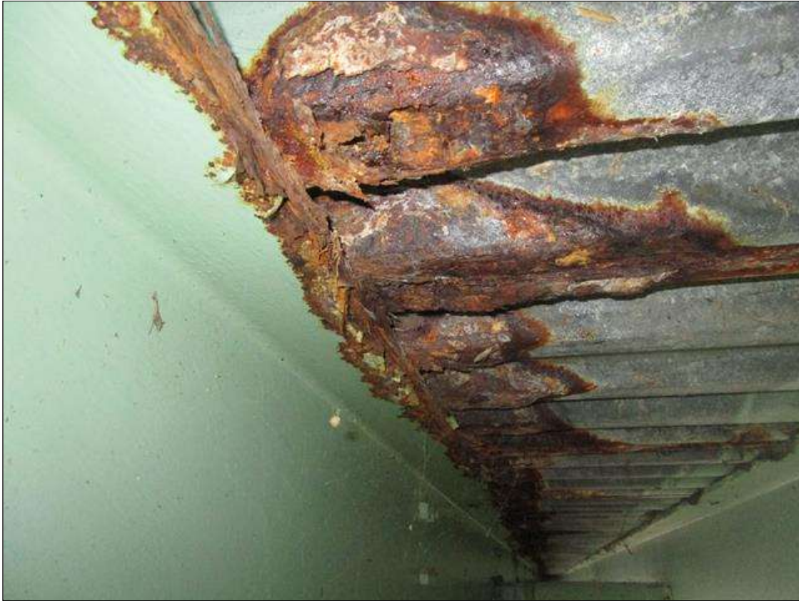
Span 4 Deck: BAY 11, DECK SOFFIT, 20FT X 1FT AREA OF 25% SECTION LOSS, PAR
