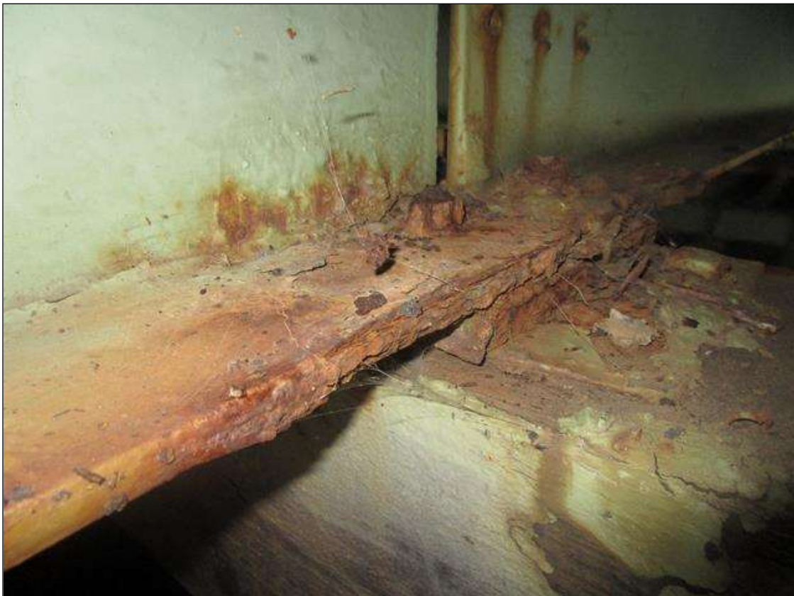
Span 5 Beam 4 - Near Bearing: ANCHOR BOLT COMPLETELY CORRODED, PAR
