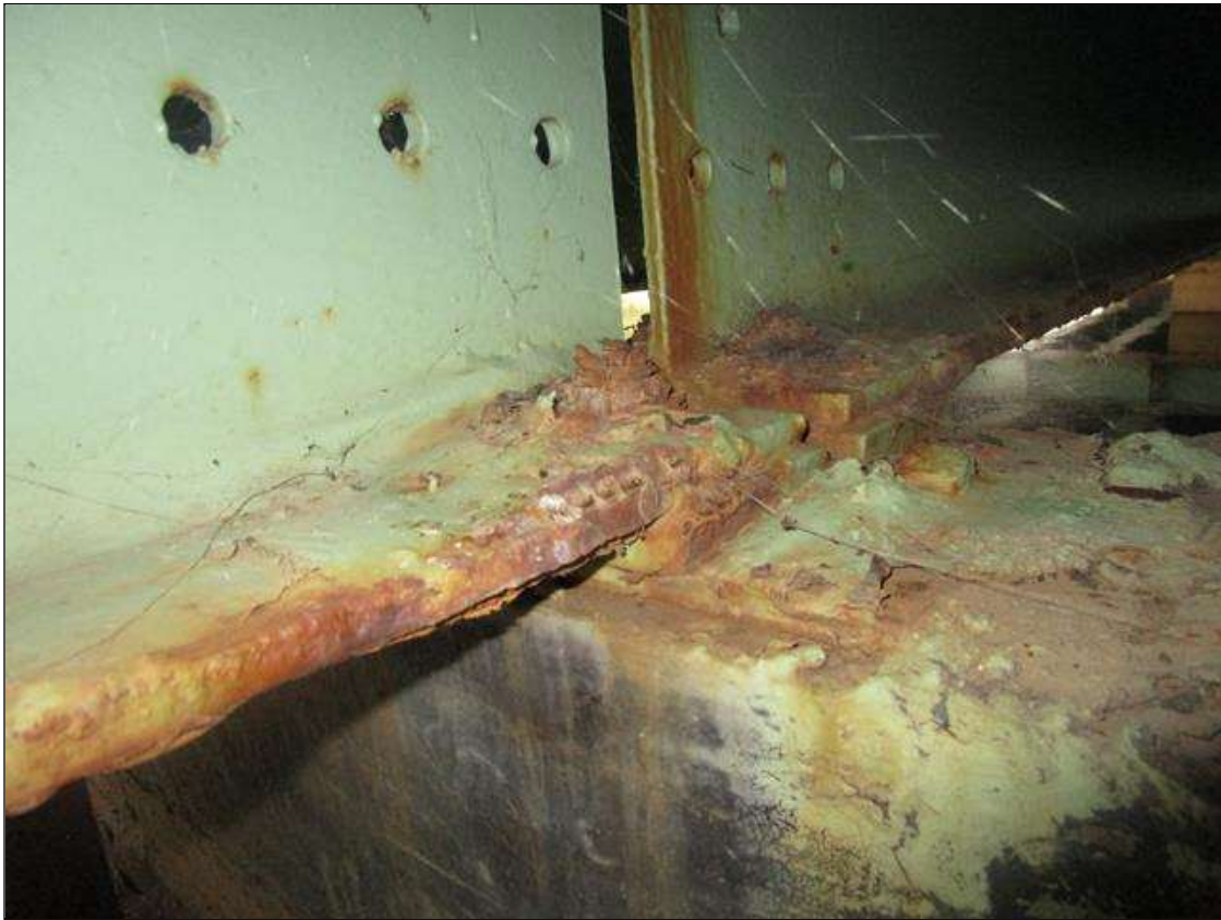
Span 5 Beam 9 - Near Bearing: ANCHOR BOLT COMPLETELY CORRODED, PAR
