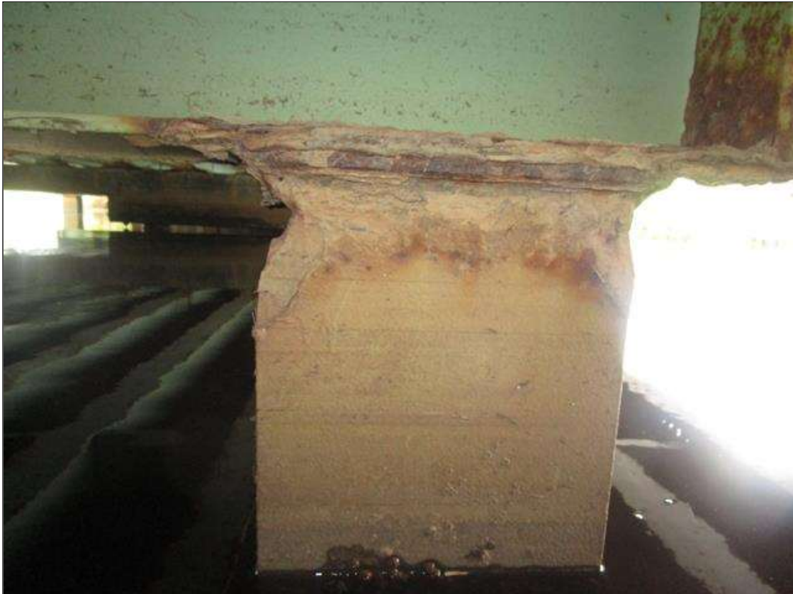
Bent 3 Pile 5: 2IN LONG X 1IN WIDE X 100% SECTION LOSS OF BOTH EDGES AT BOTH FLANGES AT TOP OF PILE. 1/8IN SECTION LOSS IN TOP PLATE, PAR
