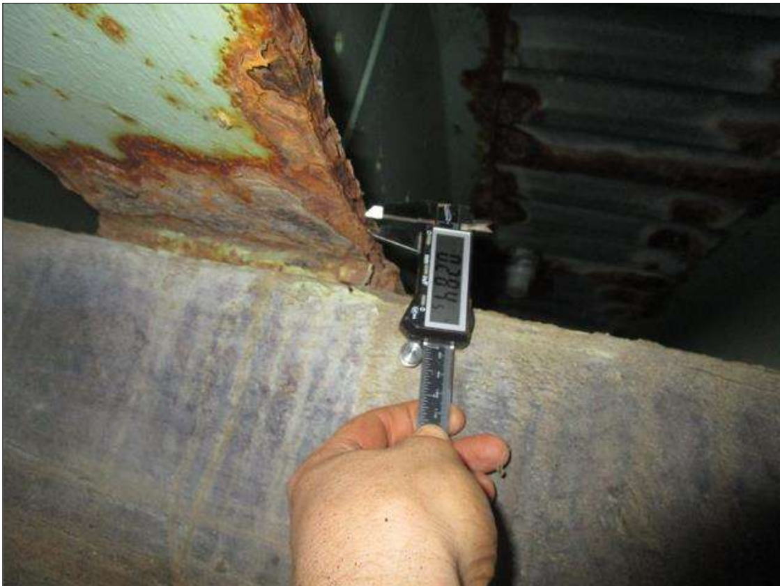
Span 3 Beam 3: SPAN 4, AT BENT 4, 1FT AREA OF SECTION LOSS DOWN TO 0.284IN REMAINING IN BOTTOM FLANGE, PAR
