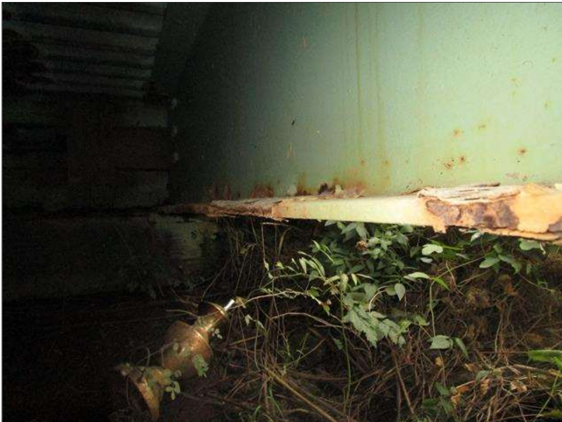
Span 1 Beam 1: SPAN 1, AT END BENT 1, 10FT INTERMITTENT AREA OF SECTION LOSS IN BOTTOM FLANGE DOWN TO KNIFE'S EDGE, PAR
