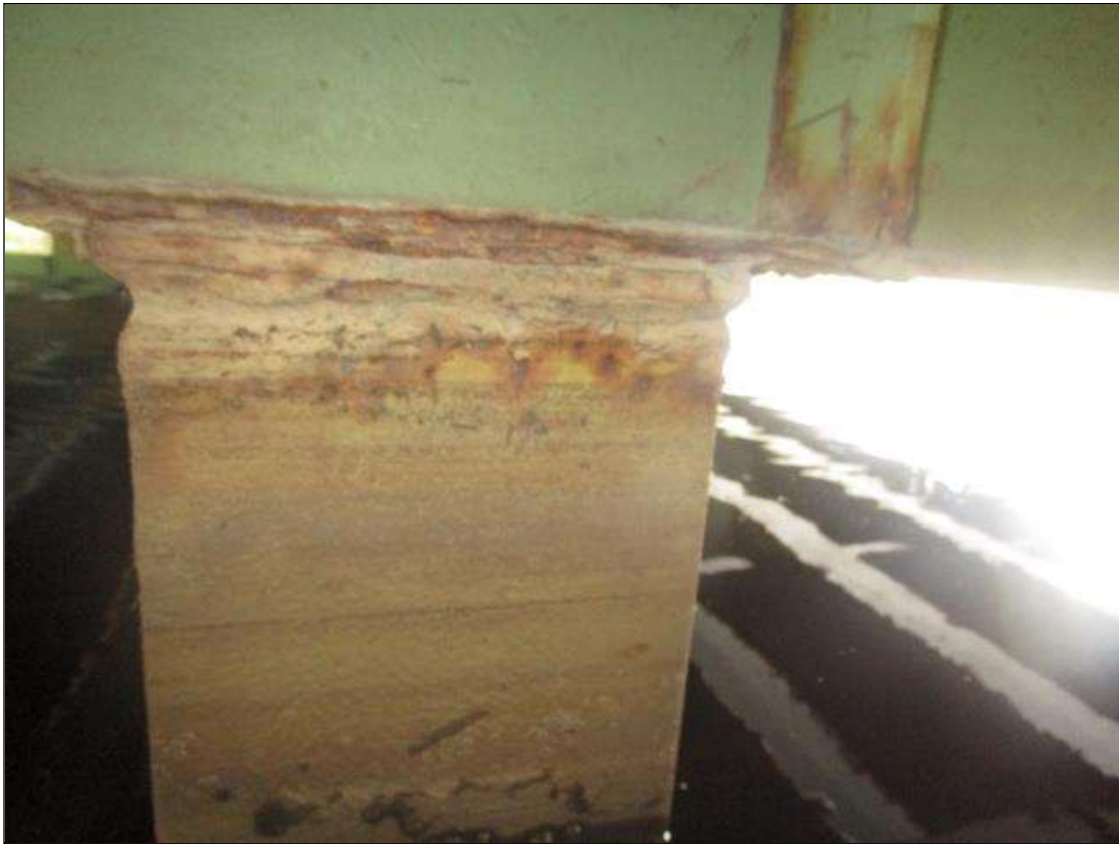
Bent 1 Pile 4: 2IN LONG X 1IN WIDE X 100% SECTION LOSS OF BOTH EDGES AT BOTH FLANGES AT TOP OF PILE. 1/8IN SECTION LOSS IN TOP PLATE, PAR
