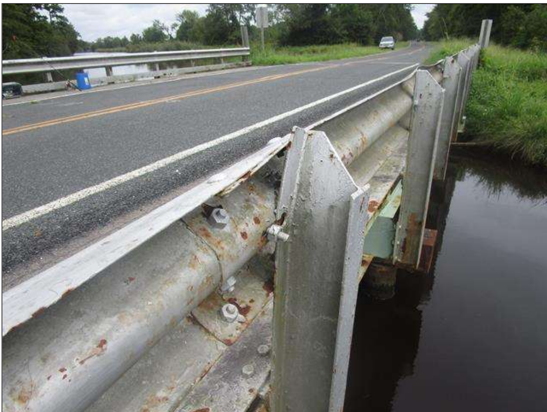
Span 4 Right Bridge Rail: BENT POST 2 WITH LOSS OF CONNECTION TO GUARD RAIL, PAR
