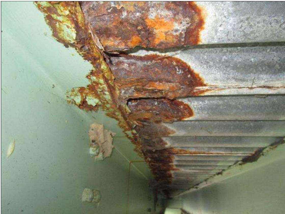
Span 5 Deck: BAY 5, 20FT X 1FT AREA OF 50% SECTION LOSS, PAR
