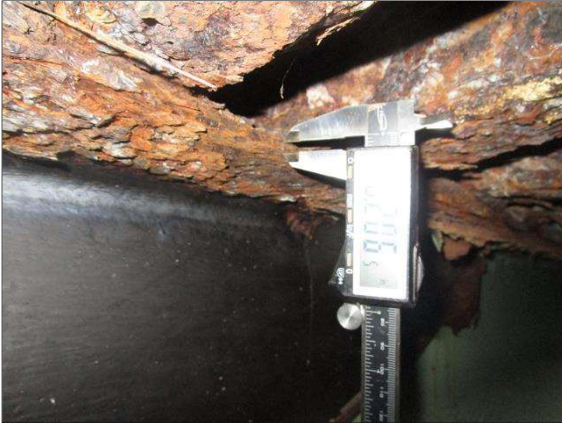
Span 5 Beam 5: SPAN 5, MIDSPAN, SECTION DOWN TO 0.206IN REMAINING IN TOP FLANGE, PAR
