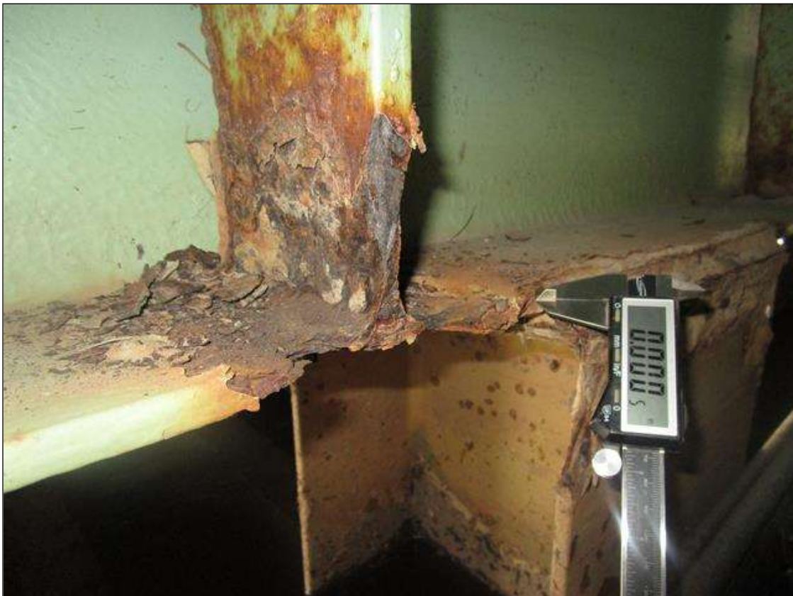
Bent 3 Cap 1: AT BEAM 3 AND PILE 2, 1IN WIDE X 100% SECTION LOSS, PAR
