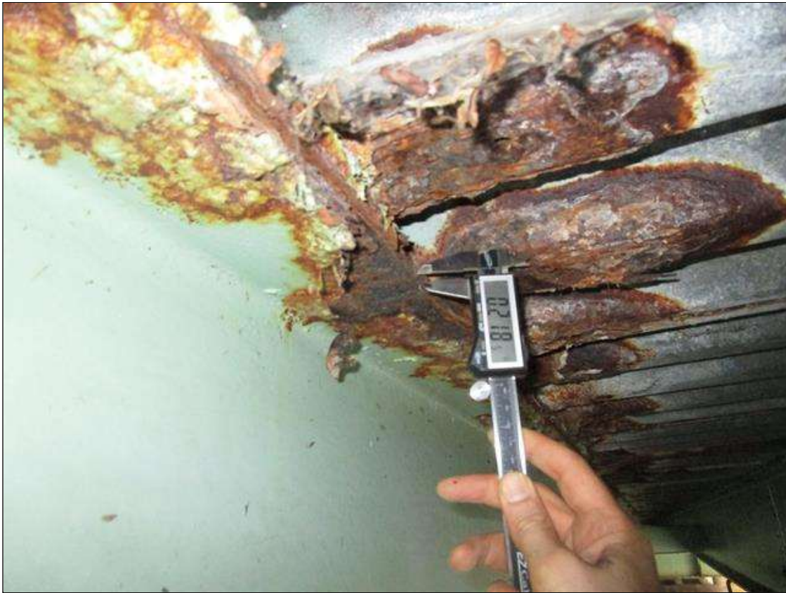
Span 5 Beam 3: SPAN 5, INTERMITTENT FULL LENGTH SECTION LOSS DOWN TO 0.218IN REMAINING, PAR
