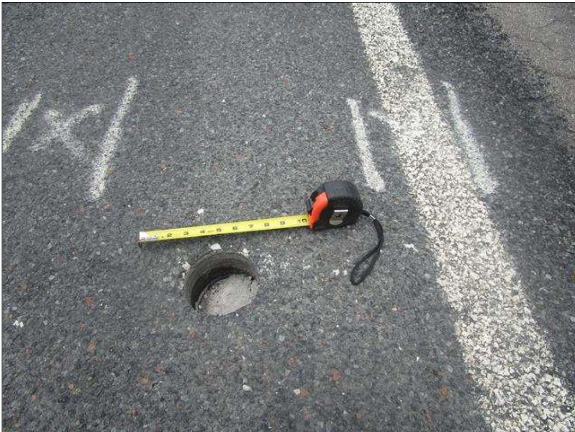
Span 2 Wearing Surface: 5FT FROM BENT 2 IN WESTBOUND LANE, 4IN DIAMETER X 4IN DEEP DIAMETER POTHOLE, PAR
