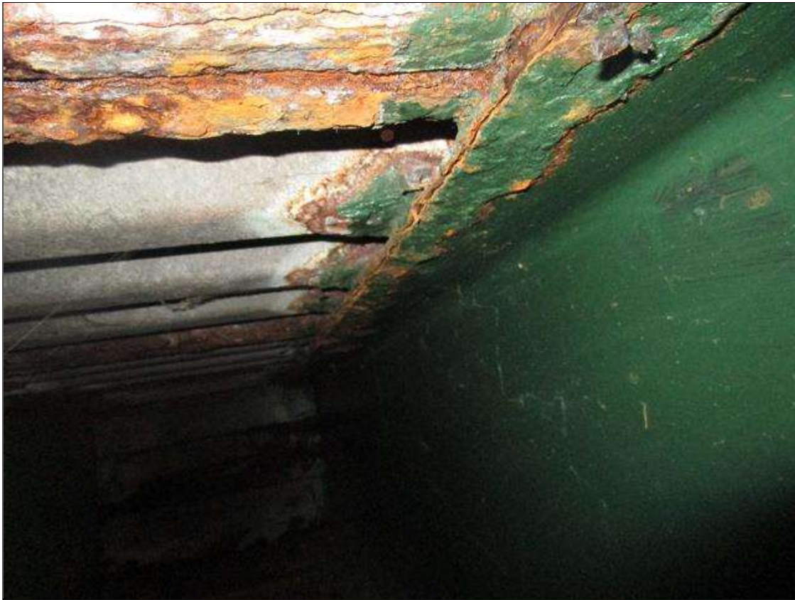
Span 1 Beam 2: SPAN 1, 7FT INTERMITTENT AREA OF SECTION LOSS DOWN TO 3/8IN REMAINING IN TOP FLANGE, PAR
