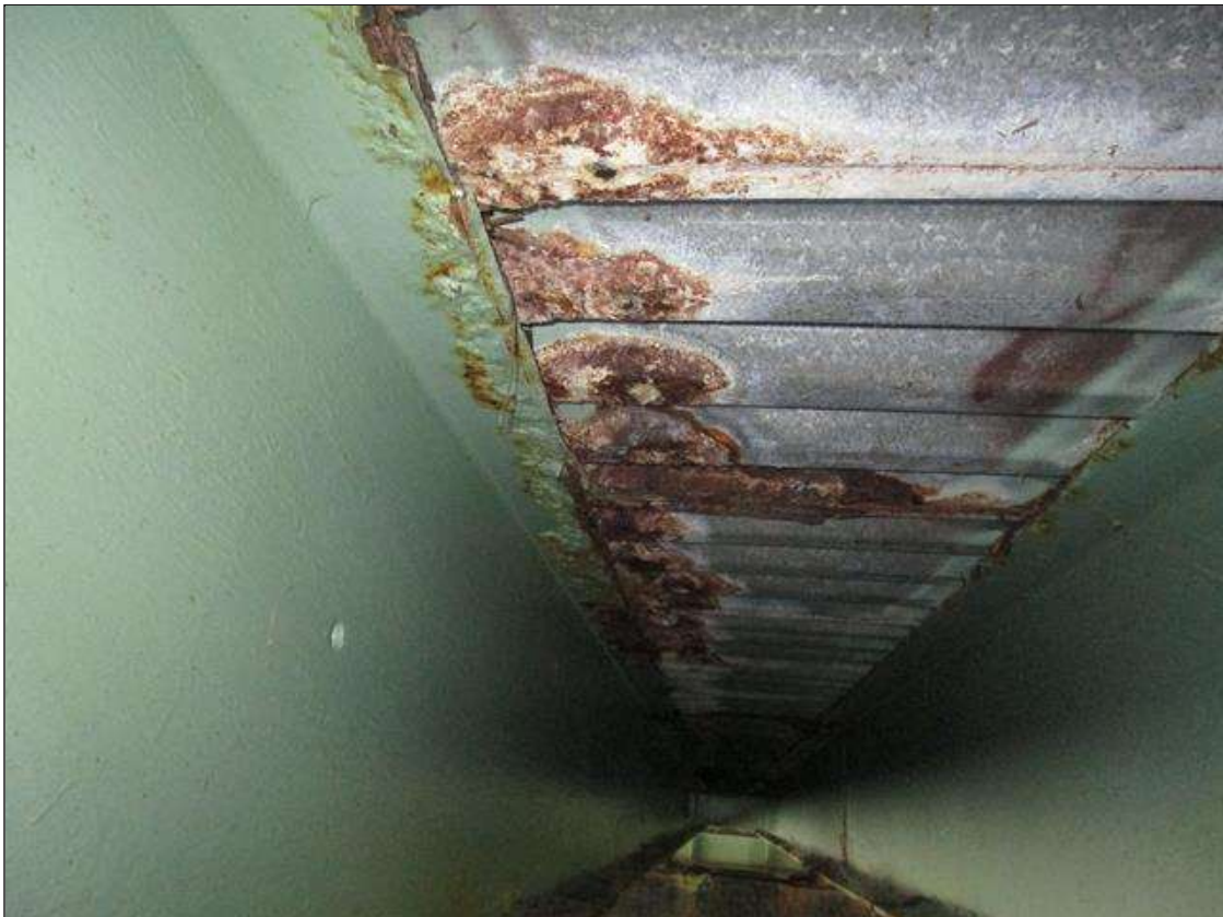
Span 5 Deck: BAY 8, 12FT X 1FT AREA WITH 25% SECTION LOSS, PAR
