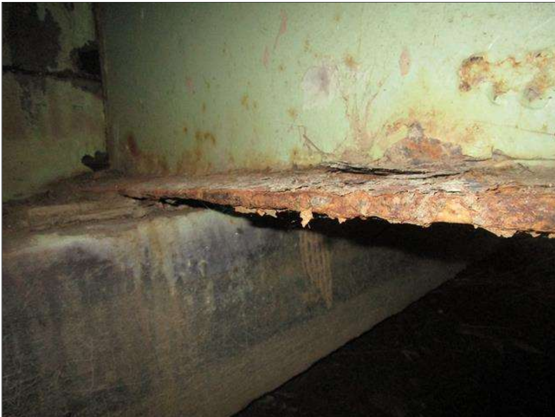
Span 1 Beam 3: SPAN 1, AT END BENT 1, 4FT AREA OF SECTION LOSS DOWN TO 1/8IN REMAINING IN BOTTOM FLANGE, PAR
