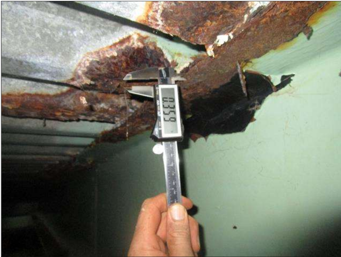
Span 3 Beam 6: SPAN 3, AT BENT 2, 3FT AREA OF SECTION LOSS IN TOP FLANGE DOWN TO 0.359IN REMAINING, PAR
