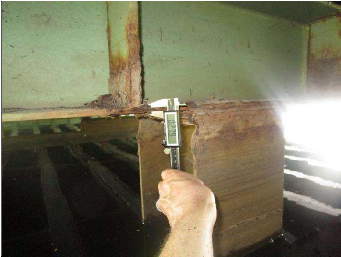
Bent 1 Cap 1: AT BEAM 5, AT PILE 3, 0.279IN REMAINING IN BOTTOM FLANGE, PAR
