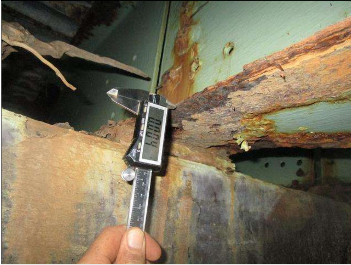
Span 3 Beam 7: SPAN 4, AT BENT 4, 2FT AREA OF SECTION LOSS DOWN TO A KNIFE'S EDGE, PAR
