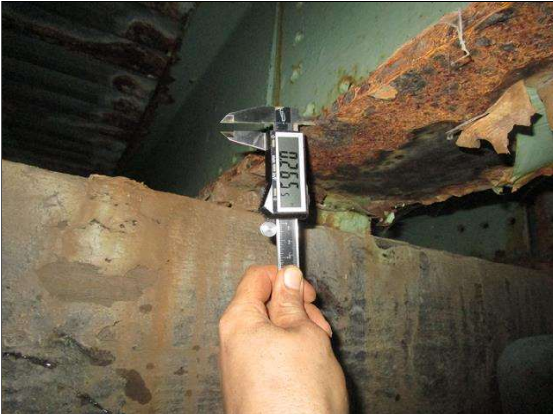
Span 1 Beam 6: SPAN 2, INTERMITTENT FULL LENGTH SECTION LOSS DOWN TO 0.265IN REMAINING IN TOP AND BOTTOM FLANGE, PAR
