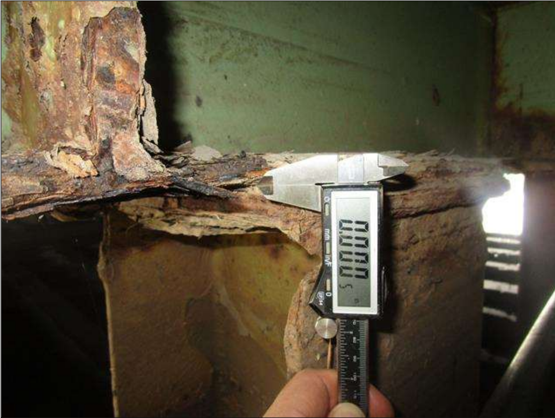
Bent 1 Cap 1: 3FT OF CORROSION IN BOTTOM FLANGE AT BEAM 3 AND PILE 2, 1IN WIDE X 1FT LONG X 100% SECTION LOSS IN EDGE OF BOTTOM FLANGE, PAR
