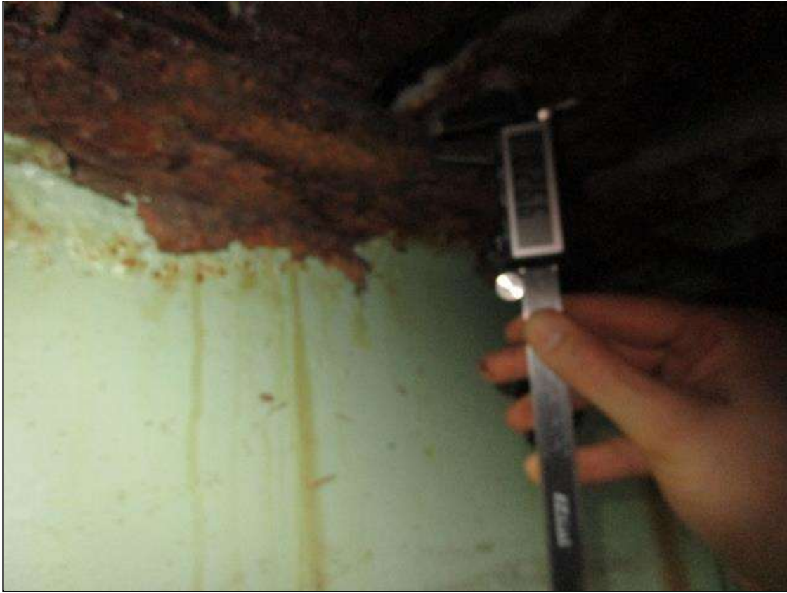
Span 5 Beam 4: SPAN 6, INTERMITTENT FULL LENGTH SECTION LOSS DOWN TO 0.266IN REMAINING IN TOP FLANGE, PAR
