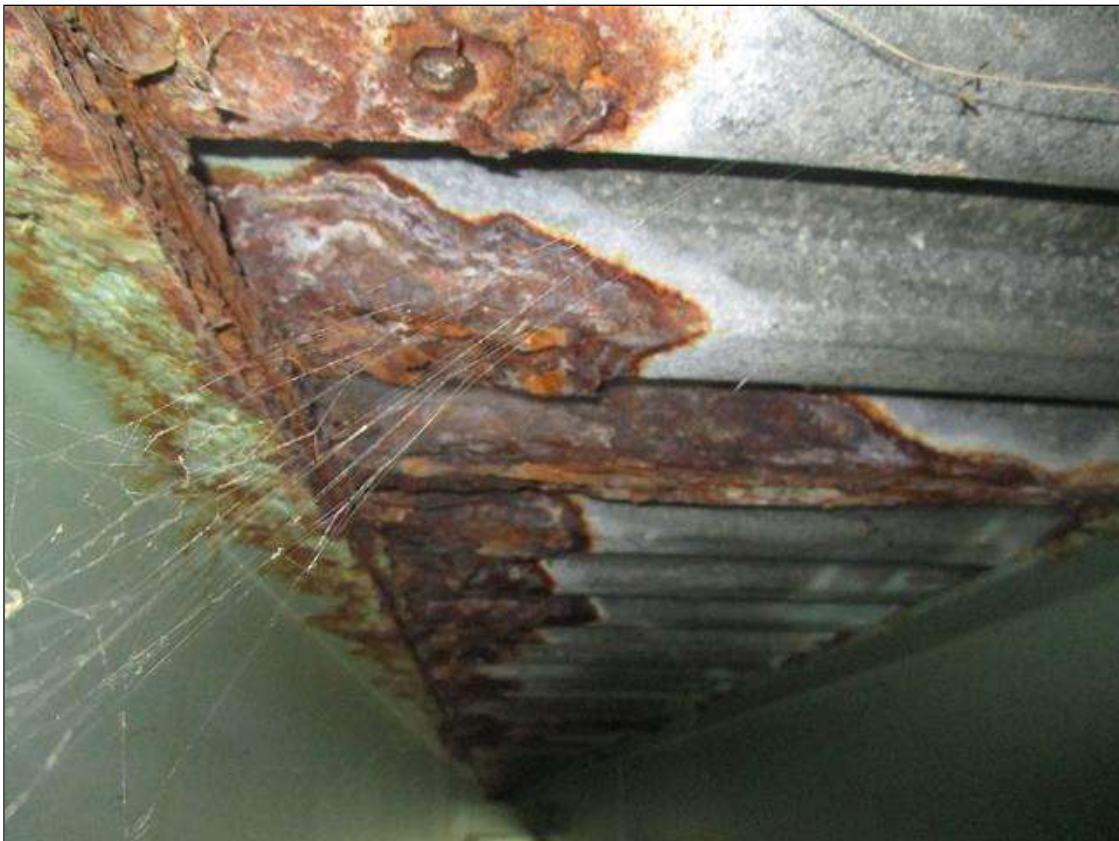
Span 5 Deck: SPAN 5 BAY 2, 10SF AREA OF SECTION LOSS DOWN TO 50%, PAR
