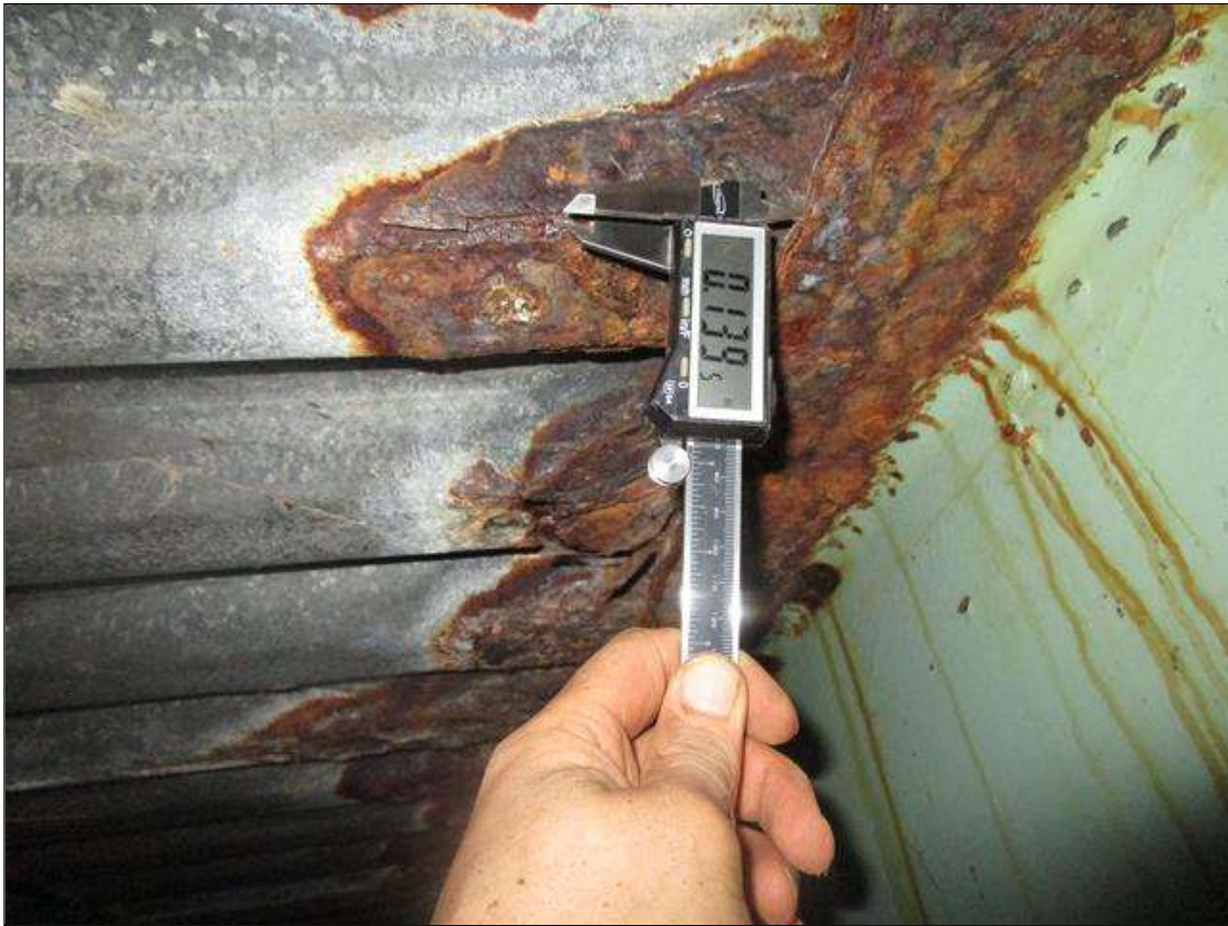
Span 1 Beam 4: SPAN 1, INTERMITTENT FULL LENGTH AREA OF SECTION LOSS DOWN TO 0.139IN REMAINING IN TOP AND BOTTOM FLANGES, PAR
