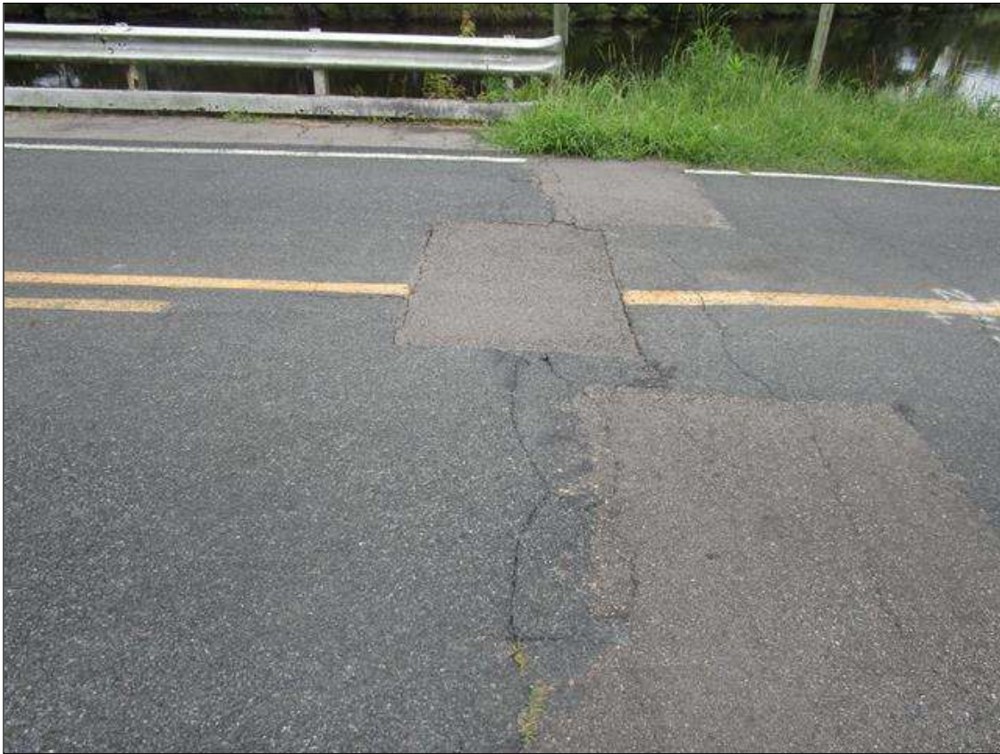
Span 6 Wearing Surface: 4' X 2' PATCHED AREA IN THE ASPHALT WEARING SURFACE AT THE CENTERLINE AT END BENT 2
