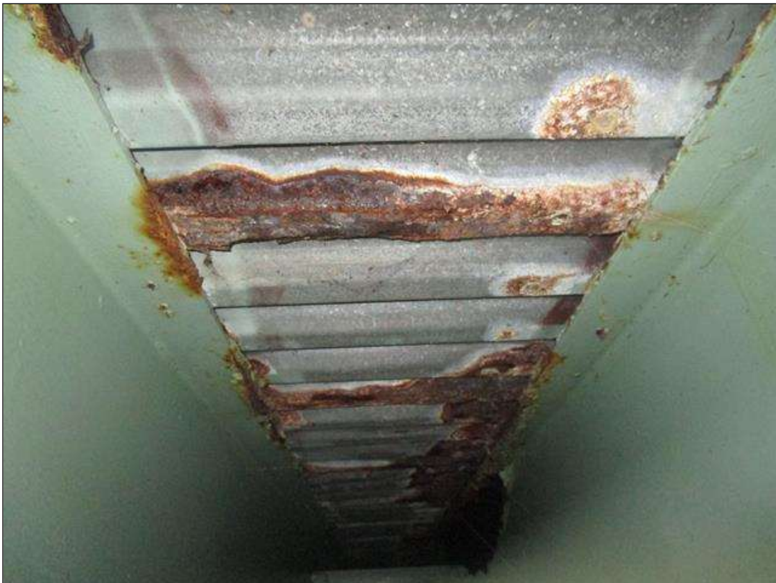
Span 5 Deck: BAY 4, 5SF AREA OF SECTION LOSS DOWN TO 25%, PAR
