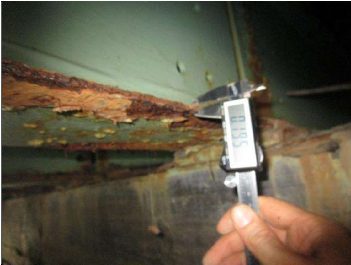
Span 5 Beam 7: SPAN 5, INTERMITTENT FULL LENGTH AREA OF CORROSION DOWN TO 0.195IN REMAINING, PAR
