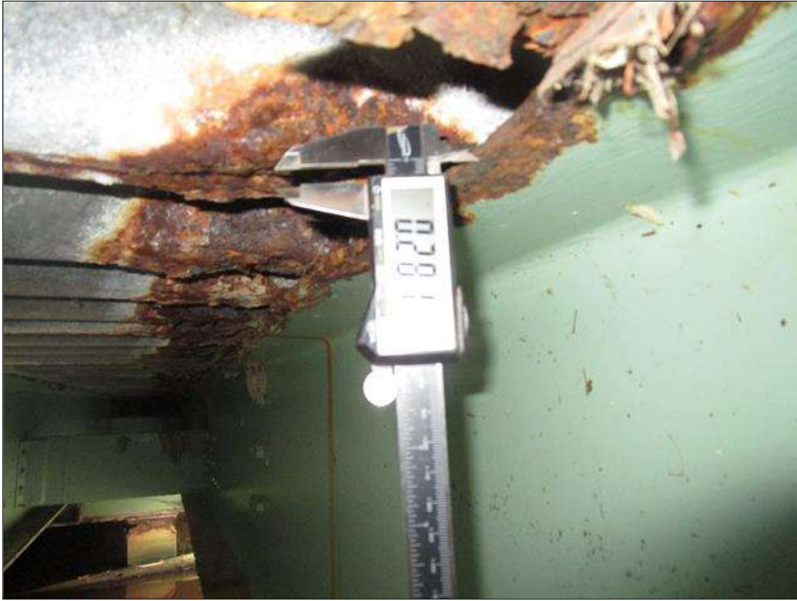
Span 5 Beam 12: SPAN 5, INTERMITTENT FULL LENGTH SECTION LOSS IN TOP AND BOTTOM FLANGES DOWN TO 0.281IN REMAINING, PAR
