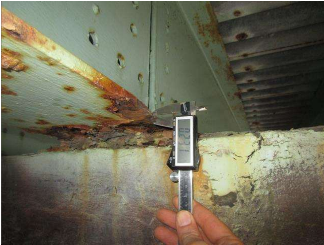
Span 5 Beam 2: SPAN 5 AT BENT 4, BOTTOM FLANGE SECTION LOSS DOWN TO 0.231IN REMAINING, PAR
