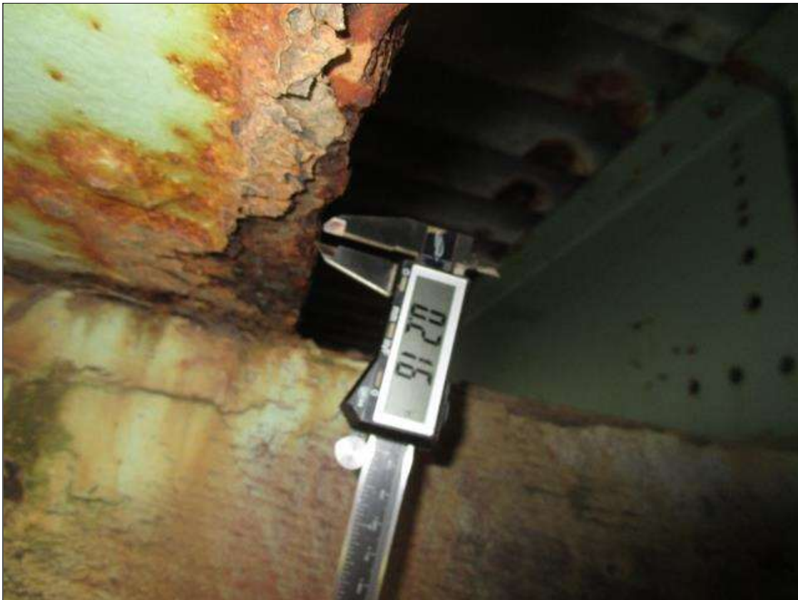
Span 3 Beam 1: SPAN 4, AT BENT 4, 1FT AREA OF SECTION LOSS DOWN TO 0.216IN REMAINING IN BOTTOM FLANGE, PAR
