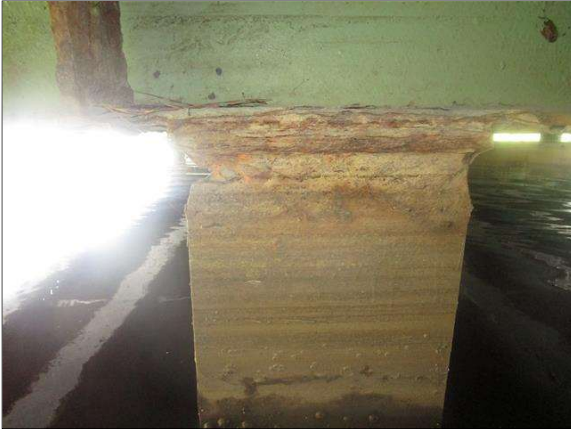
Bent 1 Pile 2: 2IN LONG X 1IN WIDE X 100% SECTION LOSS OF BOTH EDGES AT BOTH FLANGES AT TOP OF PILE. 1/8IN SECTION LOSS IN TOP PLATE, PAR
