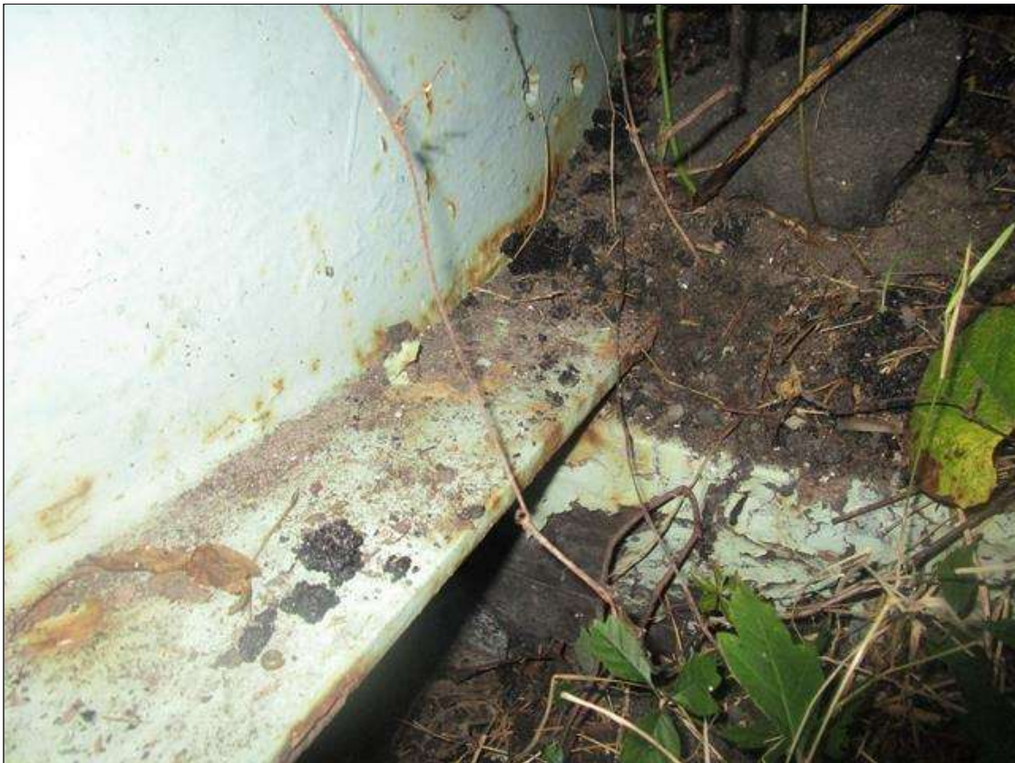
Span 5 Beam 12: SPAN 6, AT END BENT 2, 2FT AREA OF SECTION LOSS DOWN TO 5/16IN REMAINING ON BOTTOM RIGHT FLANGE, PAR
