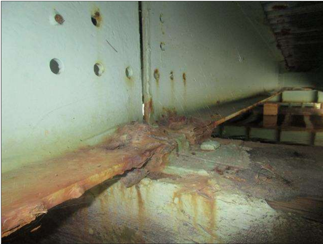
Span 5 Beam 3 - Near Bearing: ANCHOR BOLT COMPLETELY CORRODED, PAR
