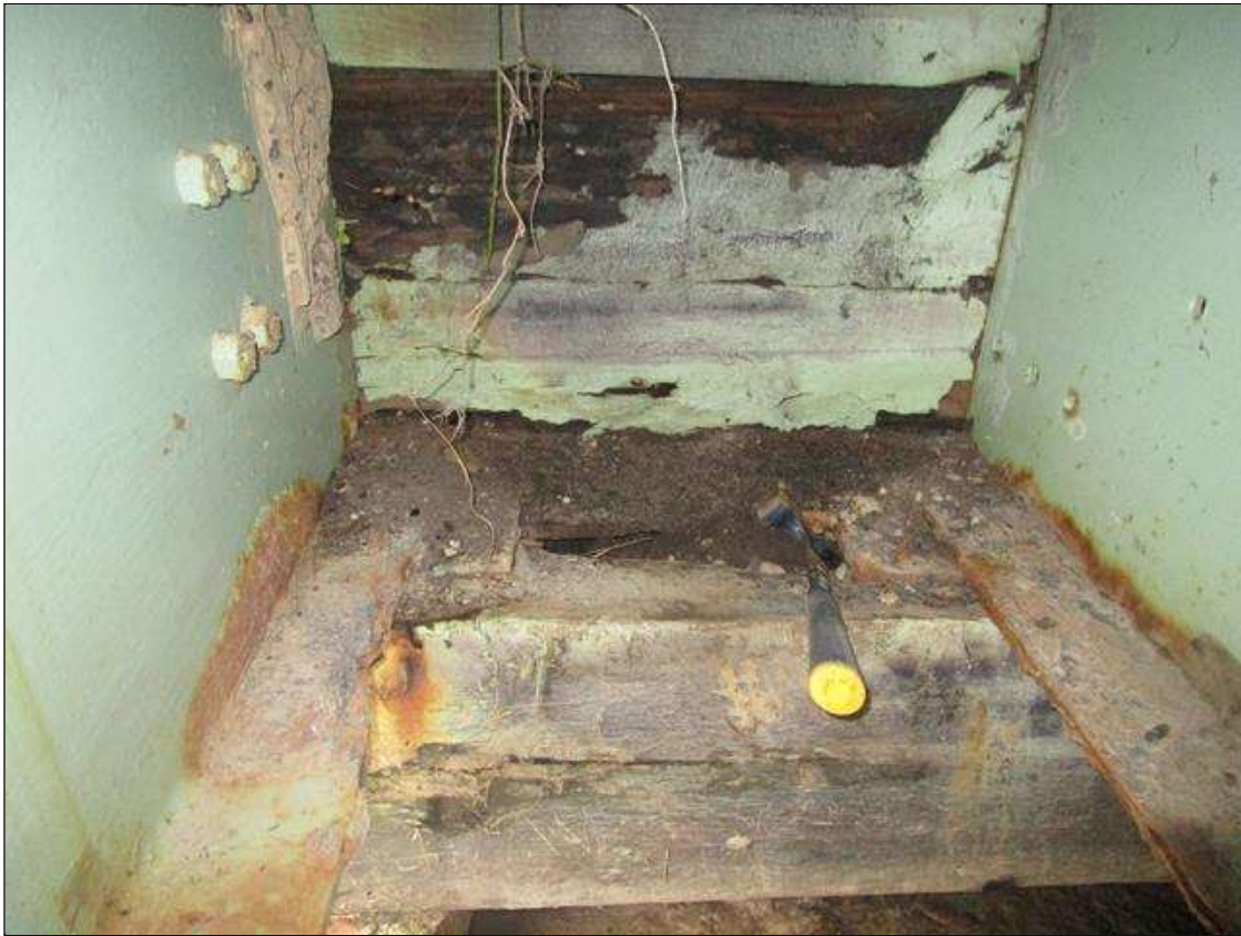
End Bent 2 Cap 1: TOP OF CAP BELOW BAYS 1-3, 6FT LONG X 8IN WIDE X 5IN DEEP DECAYED AREA. 60% LOSS OF BEARING AREA AT BEARINGS 1-3, PAR
