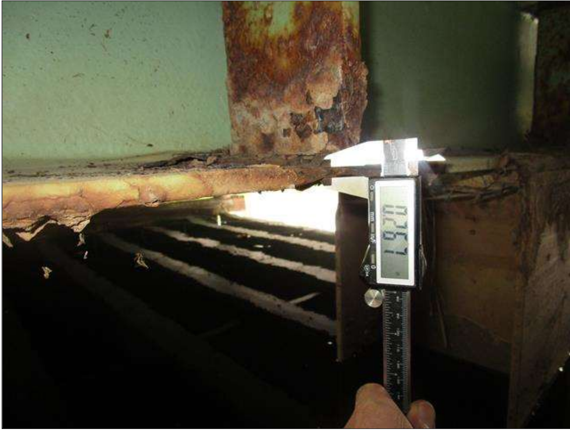
Bent 3 Cap 1: AT BEAM 7, 1FT AREA OF SECTION LOSS IN BOTTOM FLANGE DOWN TO 0.267IN REMAINING, PAR
