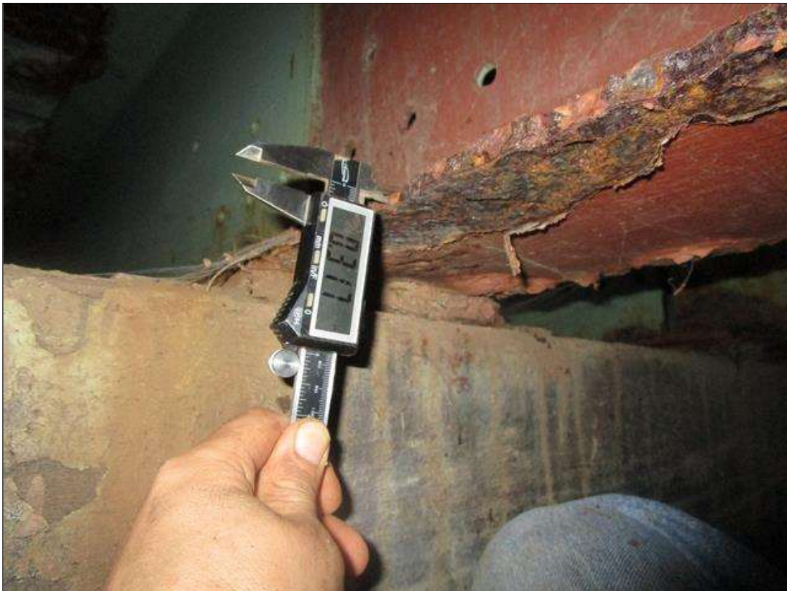
Span 1 Beam 4: SPAN 2, AT BENT 2, SECTION LOSS DOWN TO 0.317IN REMAINING IN THE BOTTOM FLANGE, PAR
