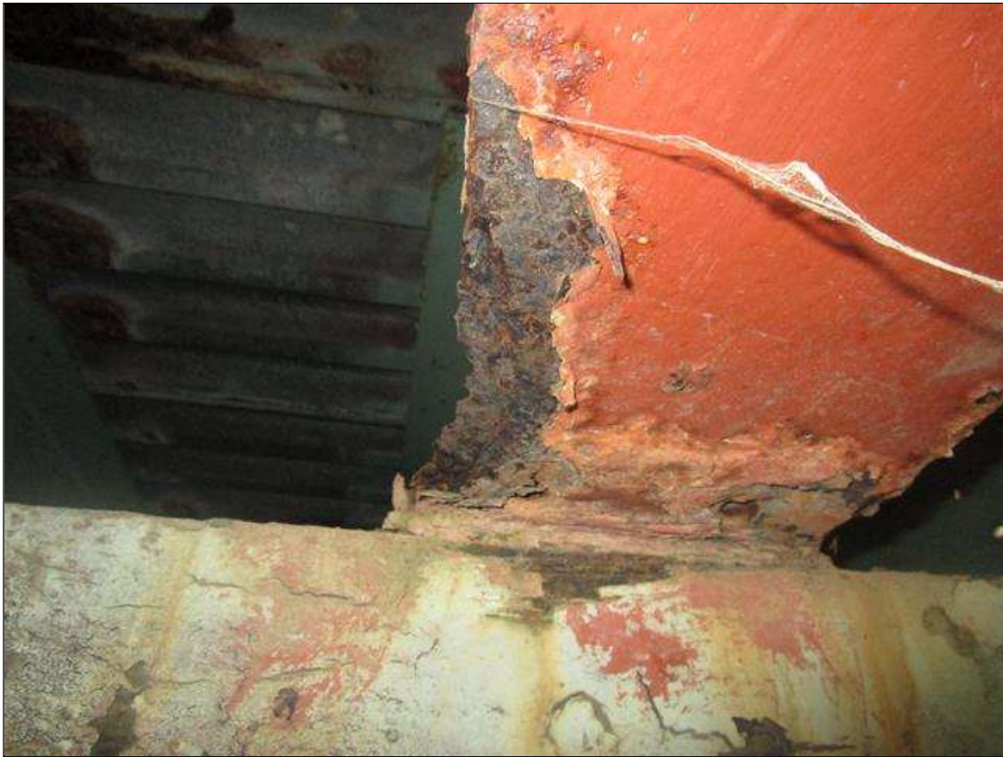
Span 3 Beam 2: SPAN 3, AT BENT 2, 1FT X 1IN WIDE AREA OF 100% SECTION LOSS IN BOTTOM FLANGE, PAR
