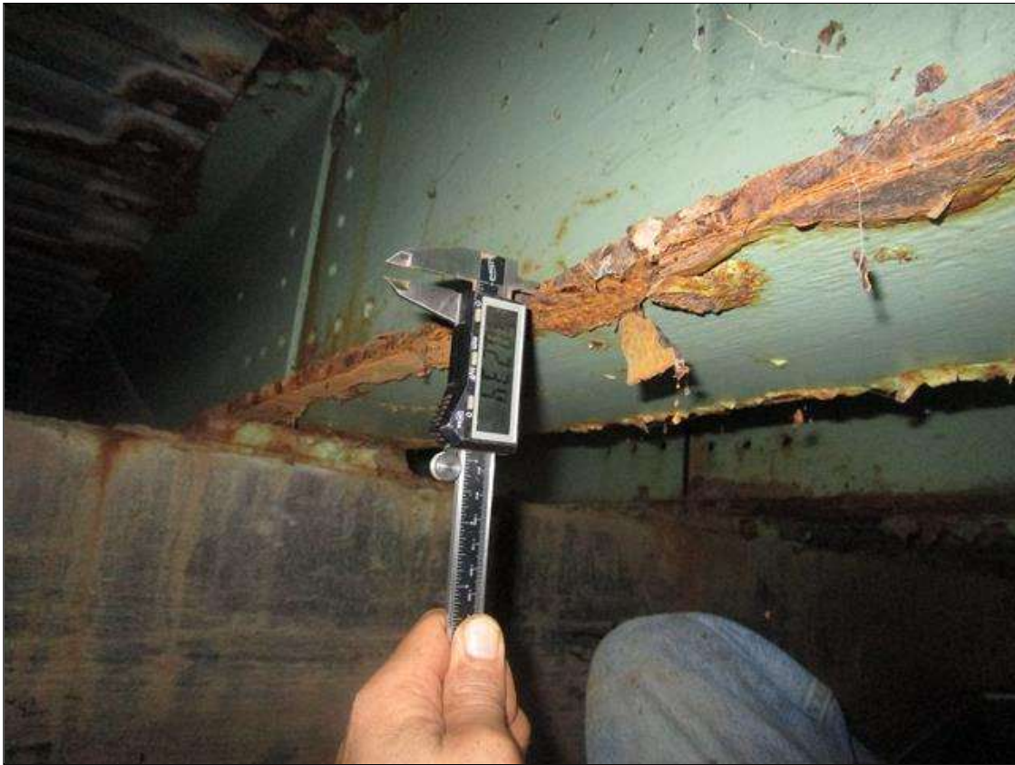
Span 1 Beam 5: SPAN 2, INTERMITTENT FULL LENGTH, 4FT AREA OF SECTION LOSS DOWN TO 0.234IN REMAINING IN TOP AND BOTTOM FLANGE, PAR
