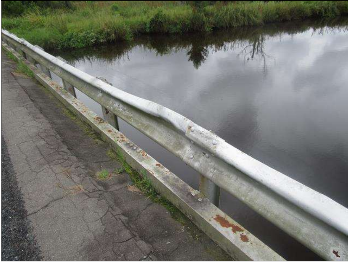
Span 2 Right Bridge Rail: AT BENT 2, 8FT LONG X 3IN DEEP IMPACT DAMAGE TO BRIDGE RAIL
