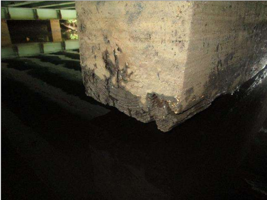
Bent 4 Cap 2: NORTH END OF SUBCAP AT PILE 3, 3IN HIGH X 12IN WIDE X 12IN DEEP DECAY, PAR
