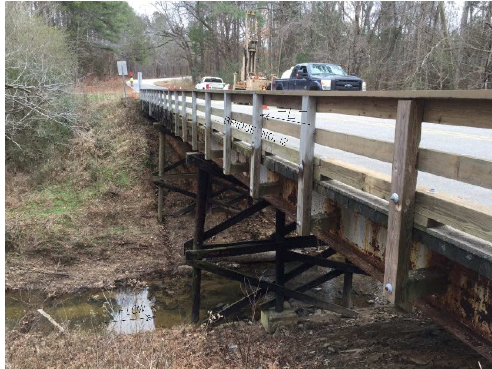
PHOTOGRAPH NO. 1: VIEW OF BRIDGE NO. 12 LOOKING EAST FROM END BENT NO. 1.
