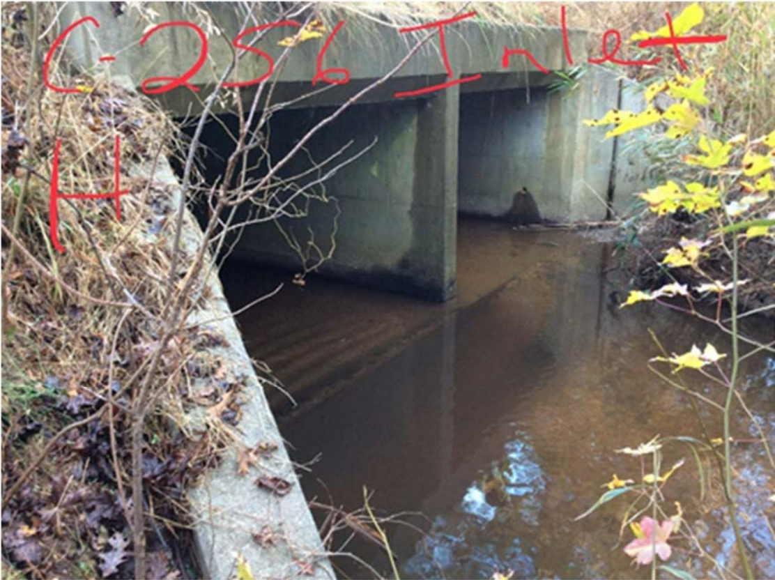
Repair Inlet toe wall scour and SE wing at barrel 1: 25' x 2' x 4' with Class II Rip Rap..
