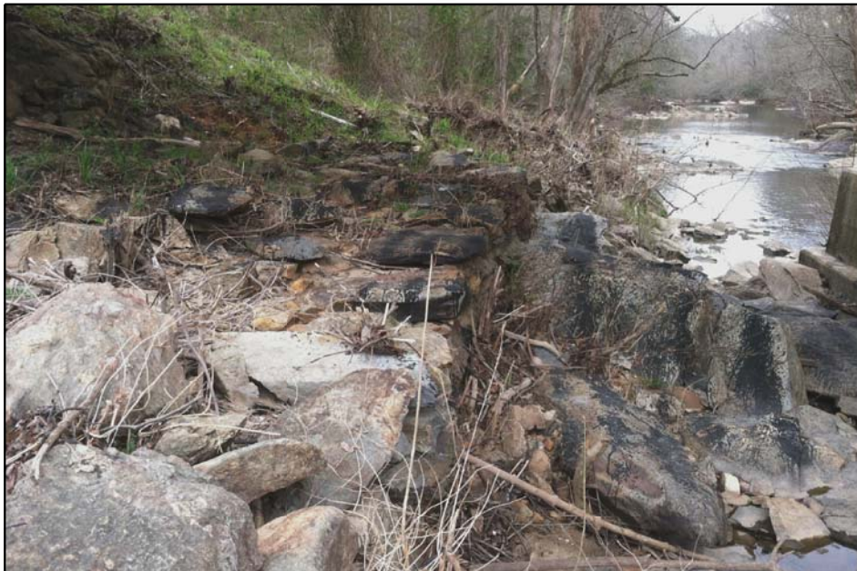
PHOTOGRAPH TAKEN FROM UNDERNEATH EXISTING BRIDGE LOOKING AT BEDROCK CONDITIONS NEAR INTERIOR BENT 2.
