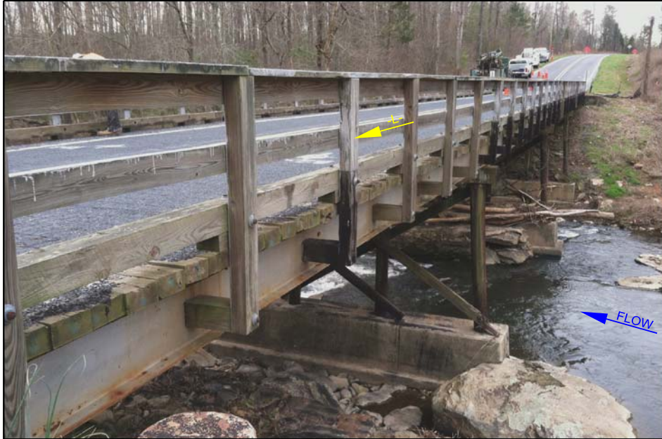
PHOTOGRAPH TAKEN FROM NEAR END BENT 2 LOOKING DOWNSTATION AT EXISTING BRIDGE STRUCTURE
