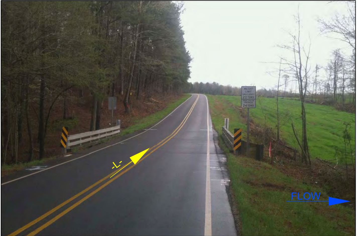
PHOTOGRAPH TAKEN FROM NEAR END BENT 1 LOOKING UPSTATION AT EXISTING BRIDGE STRUCTURE
