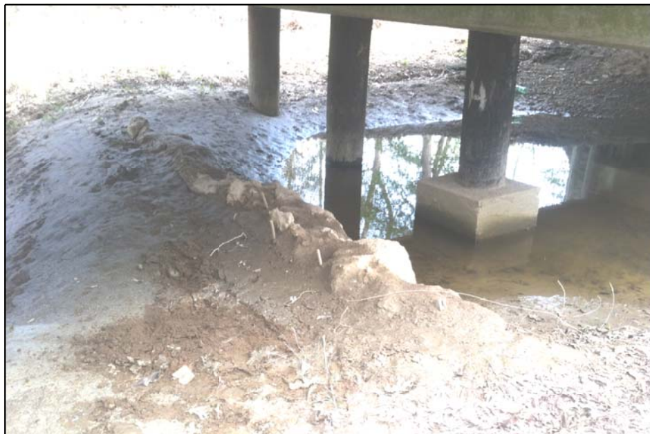
PHOTOGRAPH TAKEN FROM UNDERNEATH EXISTING BRIDGE LOOKING AT OLD BRIDGE BENT FOUNDATION.
