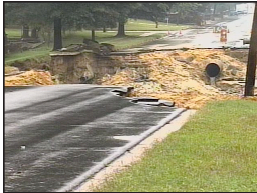
Road washout from heavy rainfall event.
