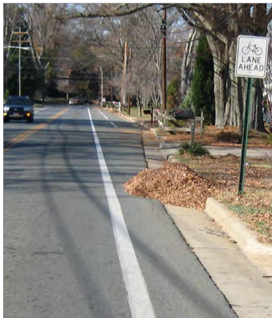
Left: Bicycle lanes on Concord Road have several maintenance issues, including yard waste in bicycle lanes and uneven pavement.
