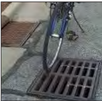
Dangerous Drainage Grate Condition; this example is dangerous due to the grate running parallel to the roadway, creating a trap for bicycle tires.
