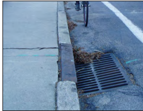
Dangerous Drainage Grate Condition; this example is dangerous due to the surrounding paving condition (when the road was resurfaced the drainage grate remained at the same height).
