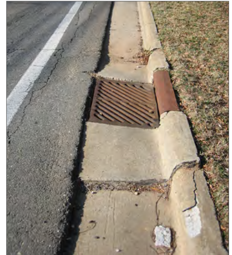
Above: An example of the uneven gutterpan/pavement seam on Concord Road, which essentially makes the functional portion of the bicycle lane less than two feet wide in some sections.
