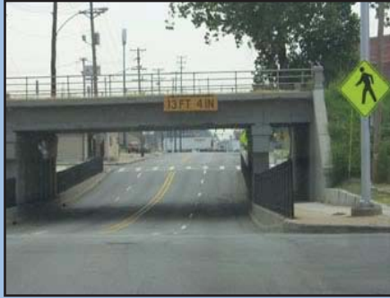
Pedestrian underpass with metal railing for pedestrian safety and separation. Photo credit: ITE Pedestrian Bicycle Council
