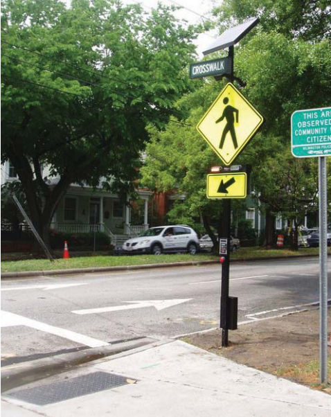
Rapid Flashing Beacon (RFB)
