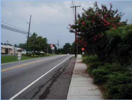
Overgrown Plants on sidewalks in downtown Hildebran provide Insufficient widths for ADA access
