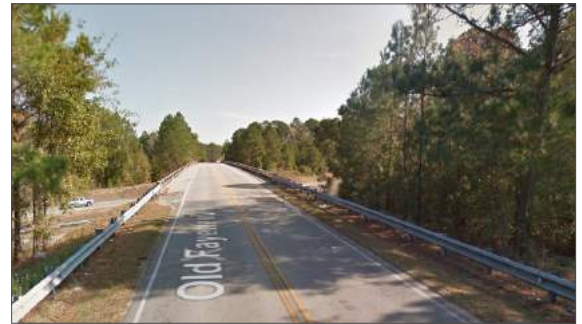
Although there are not sidewalks, school children can often be seen walking along the Old Fayetteville Street bridge over US 74.
