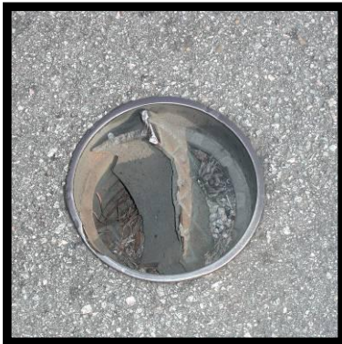
Broken utility cover
