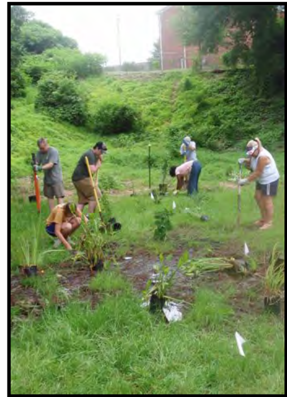
Volunteer efforts like this one to construct a rain garden require both government coordination and citizen involvement.
