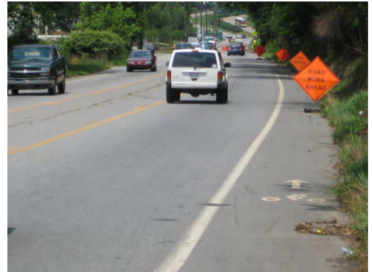
Closing a bicycle lane involves plenty of advance notice so that cyclists can merge into the main roadway.
