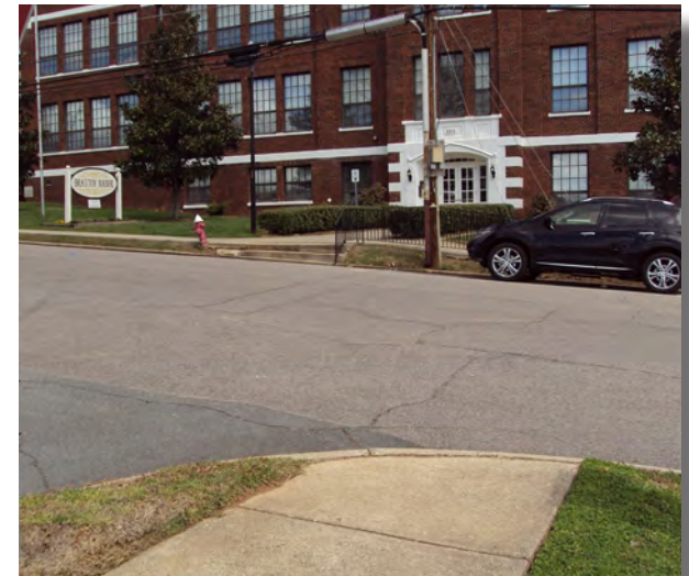
S. Third Avenue intersection without a curb ramp or crosswalk
