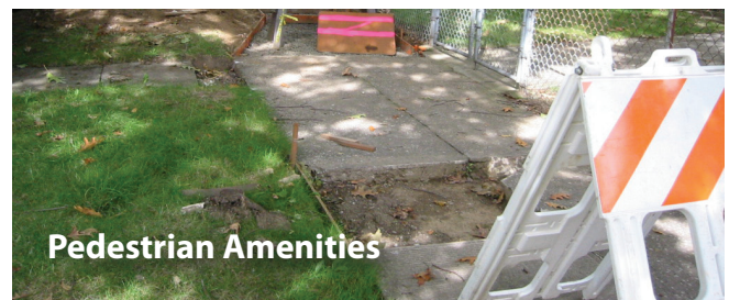
Sidewalk Obstructions and Driveway Ramps
