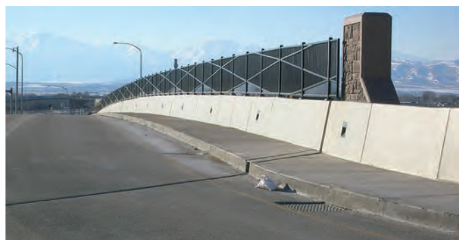
Exhibit 1-9. Sidewalk and recessed lighting located on the bridge at the Pioneer Crossing and Interstate 15 DDI (American Fork, Utah) (6).
