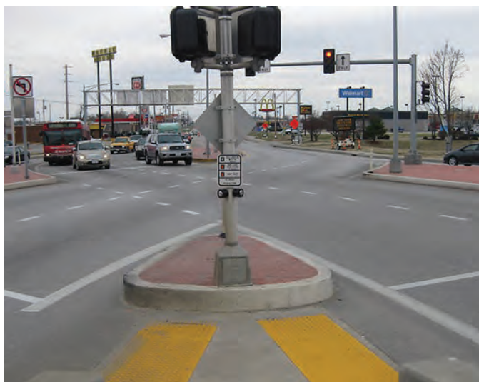
Exhibit 3-51. Undesirable use of single pole with two pedestrian push buttons, no APS, and insufficient separation of the two detectable warning surfaces (4).
