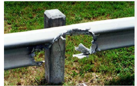
Corroded guardrail against concrete post
