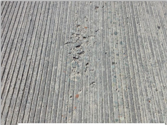
PITTED DECK SURFACE
