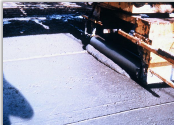
TOO MUCH CONCRETE ON DRUMS
