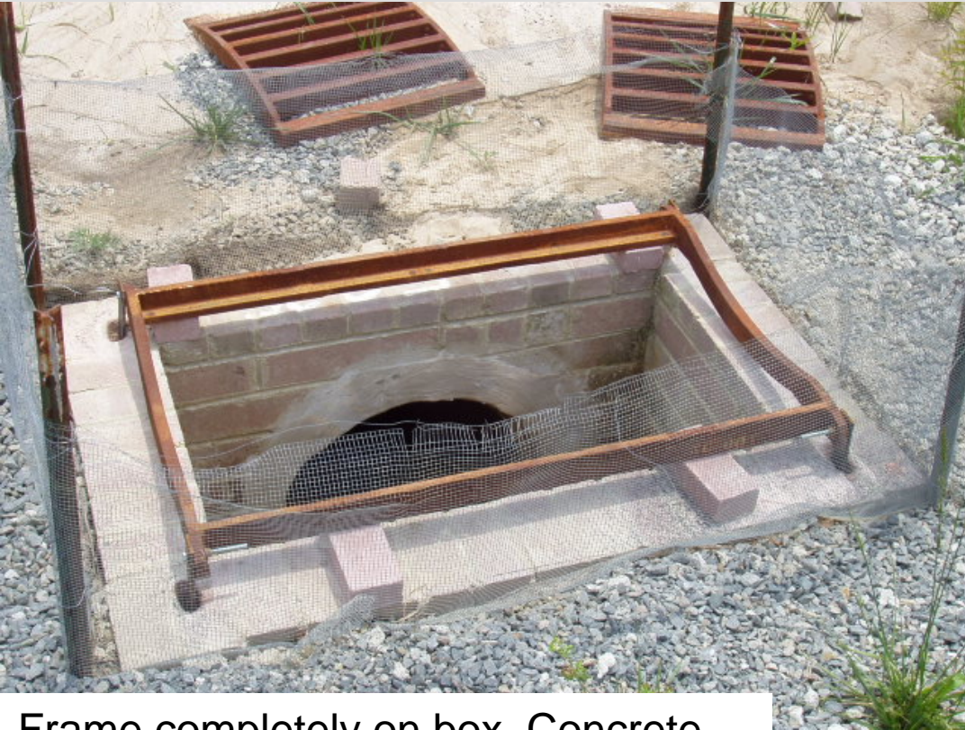
Frame completely on box. Concrete will flow under frame. Anchors in brick.
