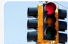
Traffic Signal TSMS
