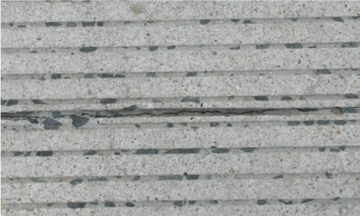
Figure 3.7 Crack in bridge deck.
