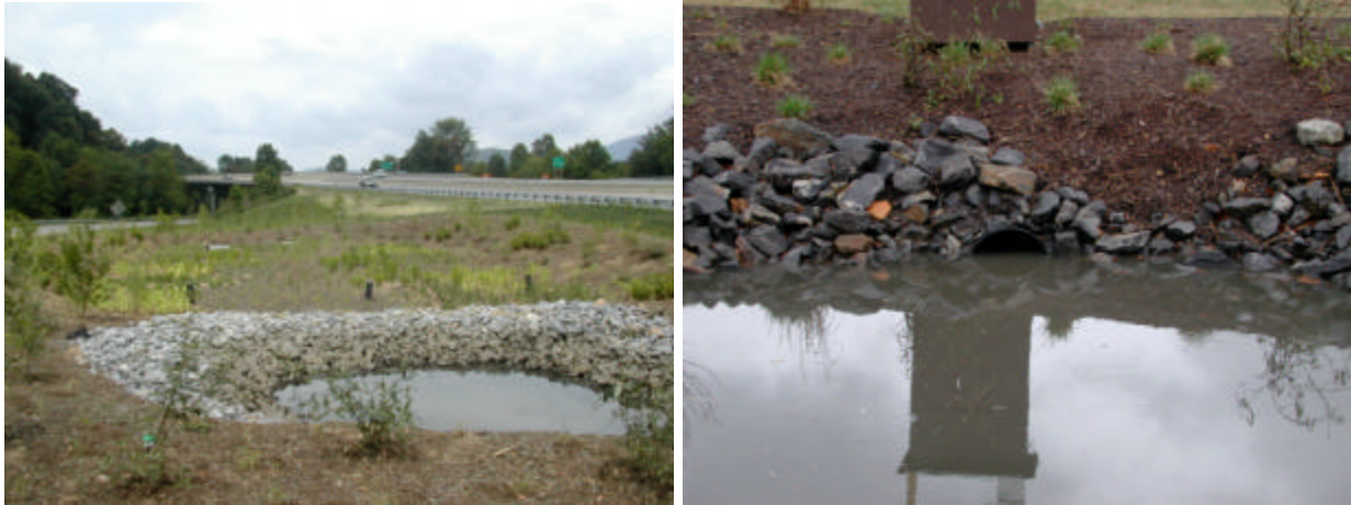
Figure 20. Division 13 bioretention area (left) and inflow pipe (right).
