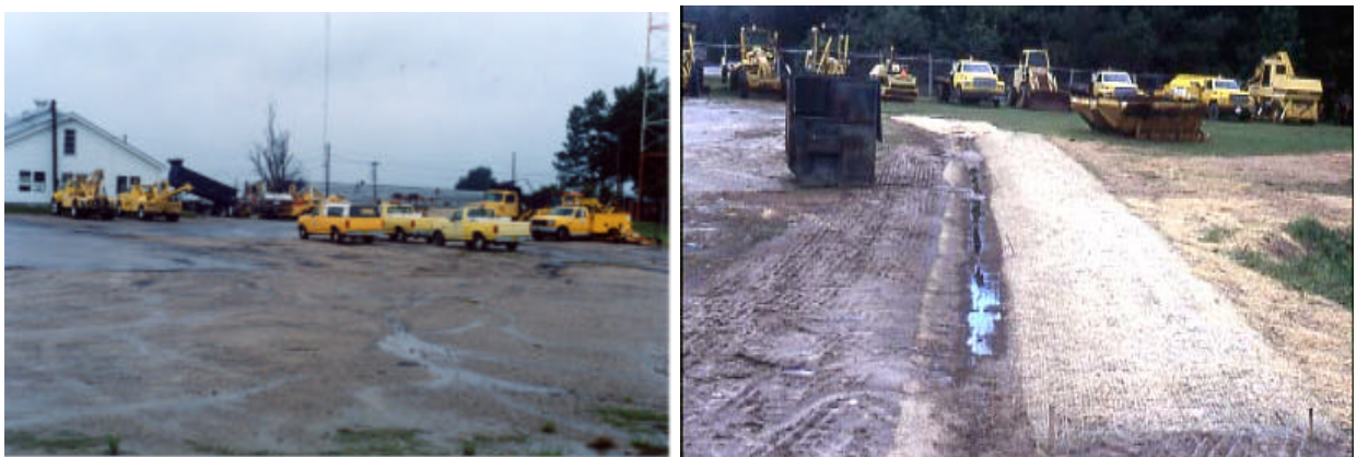
Figure 9. Lower part of the drainage (right) and diversion to carry runoff to drain inlet.
