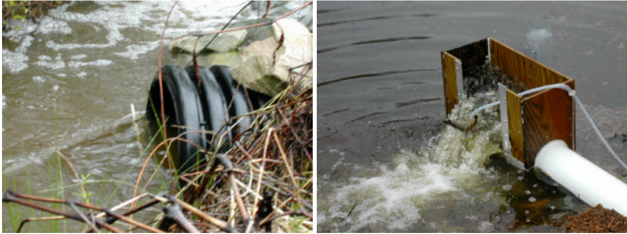
Figure 19. Ditchwater backing up into outflow pipe (left) and debris in inflow weir (right).
