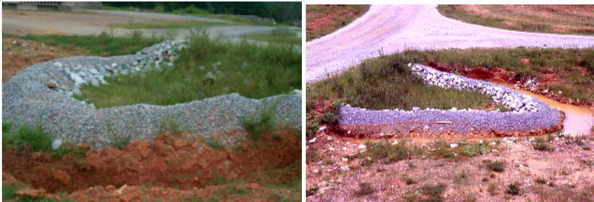
Figure 20. Sediment control device for the soil storage area of the Orange CMY.
