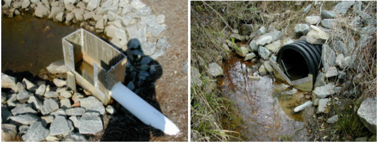
Figure 18. Inflow monitoring weir box (left) and outflow monitoring weir (right).
