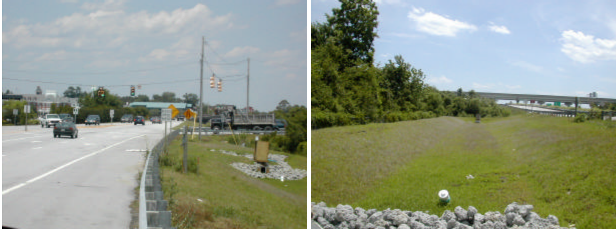
Figure 9. Part of drainage area to the swale (left) and the enhanced roadside swale (right).
