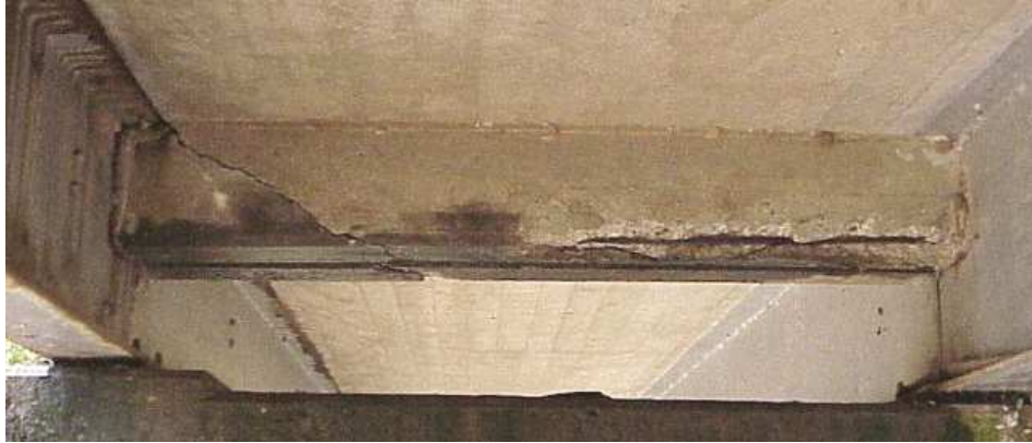
Figure 4.10 Cracked end diaphragm
