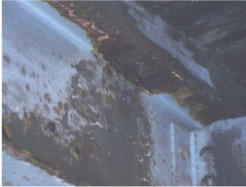
Figure 4.12 Steel girder corrosion
