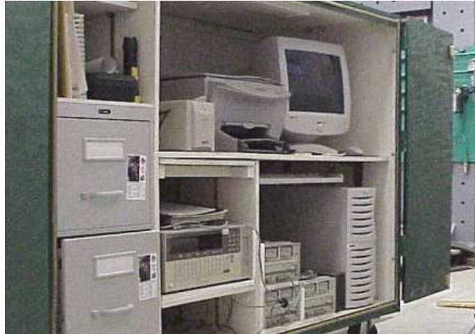
Figure C.4 Data acquisition system
