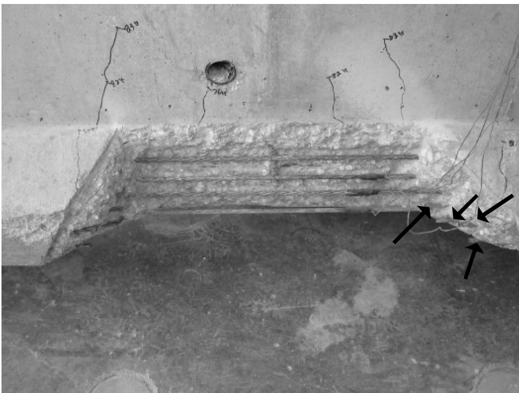
Figure 4.5 Simulated damage of AASHTO2 girder
