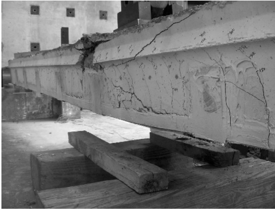
Figure 3.12 Concrete crushing failure of girder SRPF
