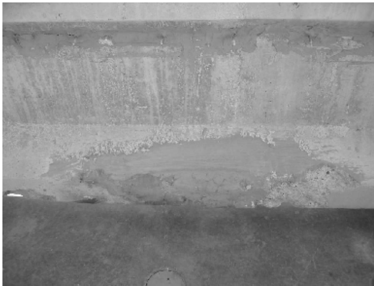
Figure 4.8 AASHTO3 defects after arriving at the testing facility
