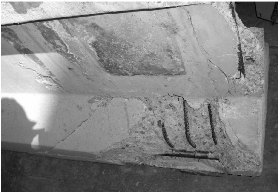
Figure 4.6 Damage to right support of AASHTO3 caused during transportation of girder
