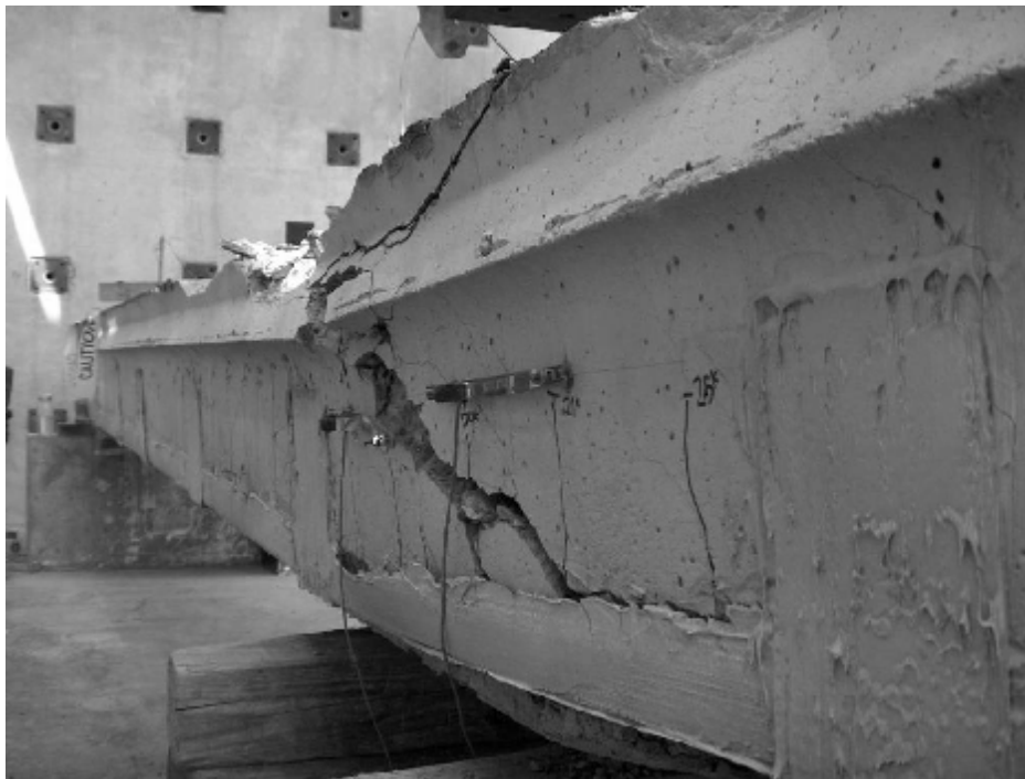
Figure 3.8 Concrete crushing failure of girder SRPS
