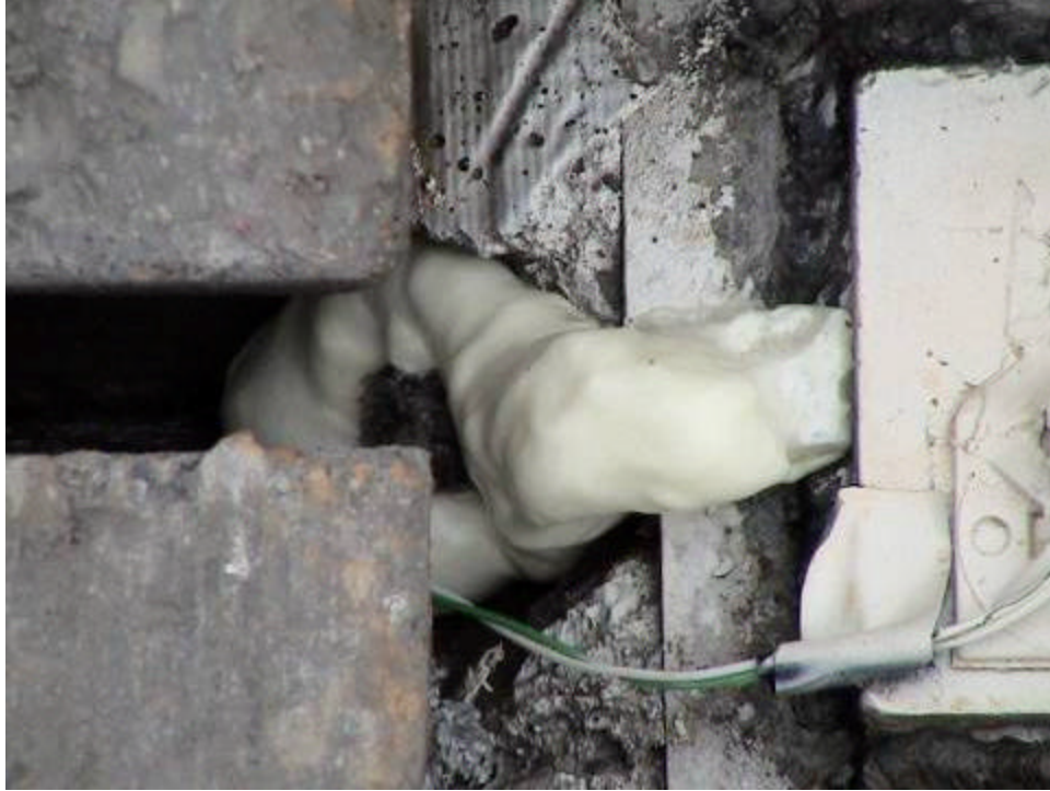
Figure A-20. Insulating Foam Used in Place of Backer Rod
