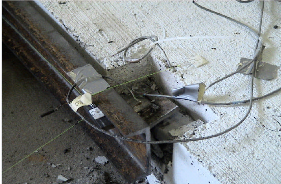
Figure 4-12. Shear Connection Failure
