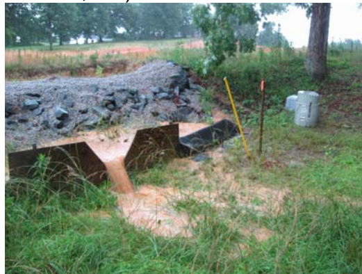
Figure 10. Standard 25-year Trap (25ST) V-notch weir with flow discharging.
