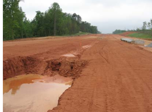
Figure 12. An estimated one ton of soil eroded from the vertical wall entrance
