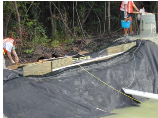
Figure 4. Rectangular weir installed to monitor flow rate discharge.
