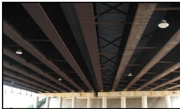
Figure 10 – Underpass SPI Lighting Mecklenburg Co., I-85 at Little Rock Rd
