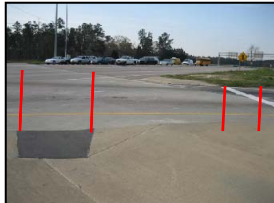
Figure 2 – Poorly Aligned Pedestrian Crossing Wake Co., I-540 at US401
