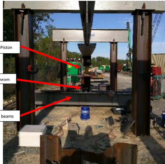
b.) Side view of reaction frame over HP 12x53 test pile with reference beams
