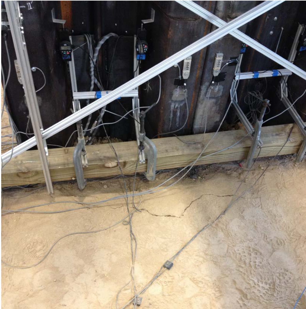
Figure 3-27: Photo showing surface cracks around the perimeter of the sheet pile wall.
