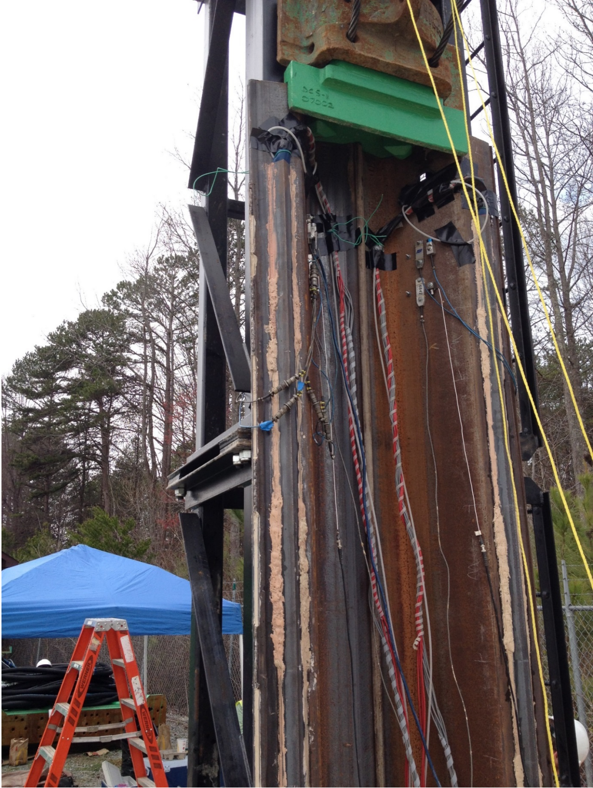
Figure B-12: Photo of PDA instrumentation on sheet piles at ICE field site.
