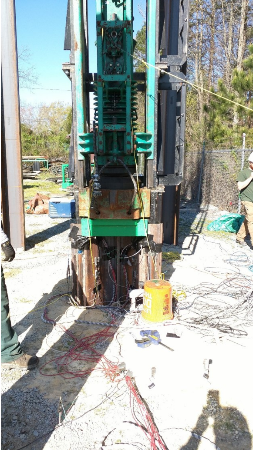
Figure B-13: Photo of PDA instrumentation on sheet piles at ICE field site.
