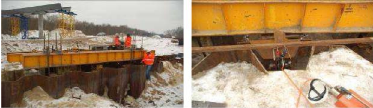
Figure 2-16: Setup of pile load test at S8 Express road in Warsaw, Poland (Skyline Steel LLC, 2009).
