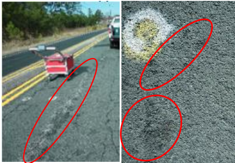
Figure 16. Images of aggregate loss problems observed at the unmodified CRS-2 field section in Durham, NC.
