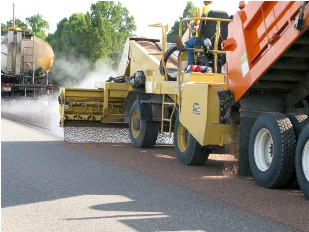
Figure A-9. Image depicting a uniform veil of chips observed from behind the aggregate spreader (Wood et al. 2006).
