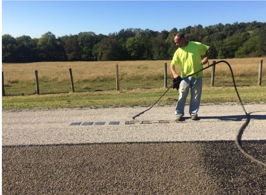
Figure 1. Construction crew patching the first chip seal layer following sample extraction and prior to applying the second layer of the double chip seal.
