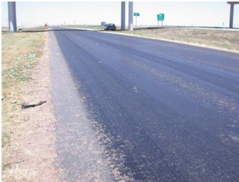
Figure A-1. Bleeding due to heavy truck traffic and hot weather (Lawson et al. 2007).
