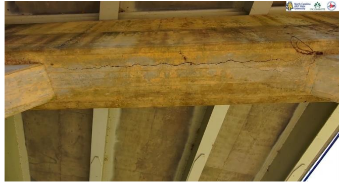
Figure 7.7: Crack on underside of pier cap, following longitudinal steel. Discoloration and staining evident from drainage.
