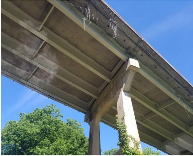
Figure 7.2 Debris pile from high flow event piled against column. Using imaging analysis technology, the volume of the pile could likely be calculated to assist in debris removal activities.
