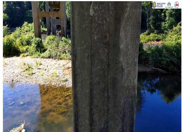
Figure 7.5: Cracks on pier over longitudinal steel. Staining evident, indicating initiation of corrosion.
