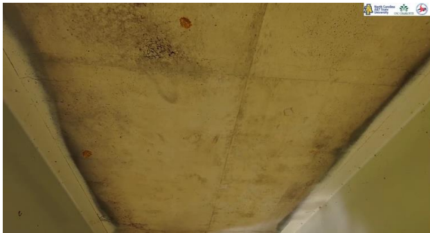
Figure 7.6 Hairline cracks visible on underside of concrete deck.
