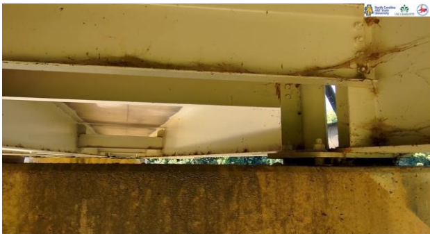
Figure 7.8: Diaphragm with bolted and welded connections shown, along with condition of concrete pier cap. Condition of bearing pad, plate, and bolts can also be observed.
