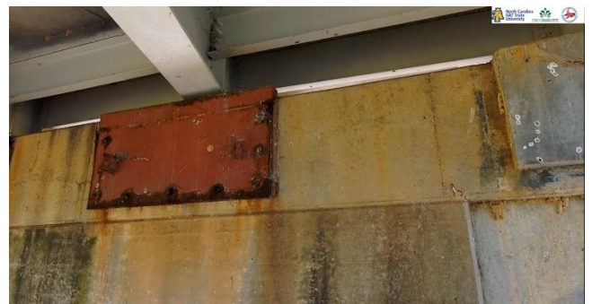
Figure 7.9: Steel plates bolted onto pier cap, with corrosion evident. Condition of girder, diaphragms and connections can also be observed.
