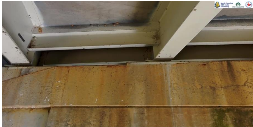
Figure 7.12: Staining and cracking in pier cap. Condition of girders and diaphragm is also evident.
