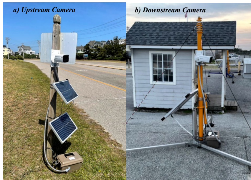
Figure 7 LPR Camera Installation: (a) Upstream LPR camera, (b) Downstream Camera
