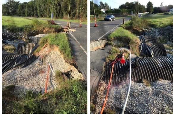
Figure 22. Photos of damage after Hurricane Florence in Site 42-1-MF.
