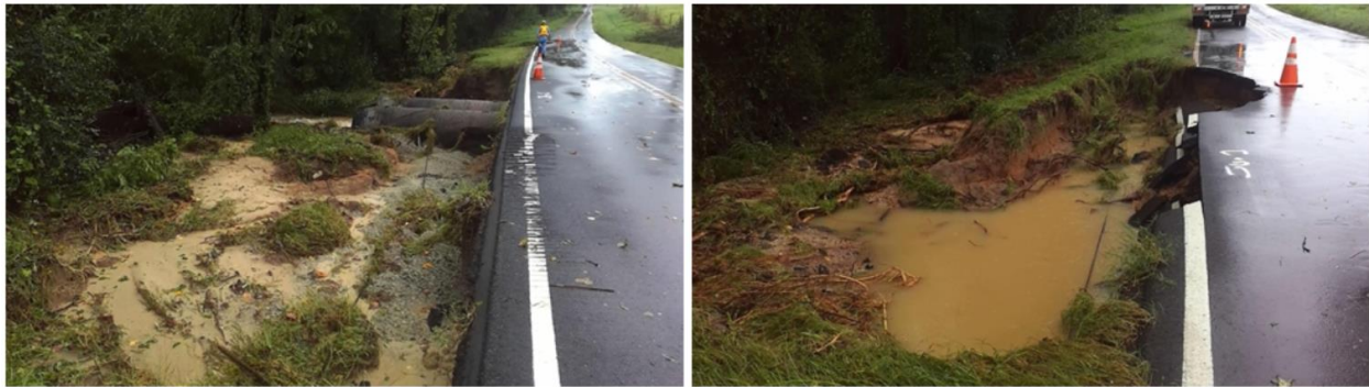
Figure 28. Photos of damage after Hurricane Florence in Site 53-4-MF.
