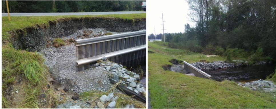
Figure 20. Photos of damage after Hurricane Florence in Site 95-4-MF.
