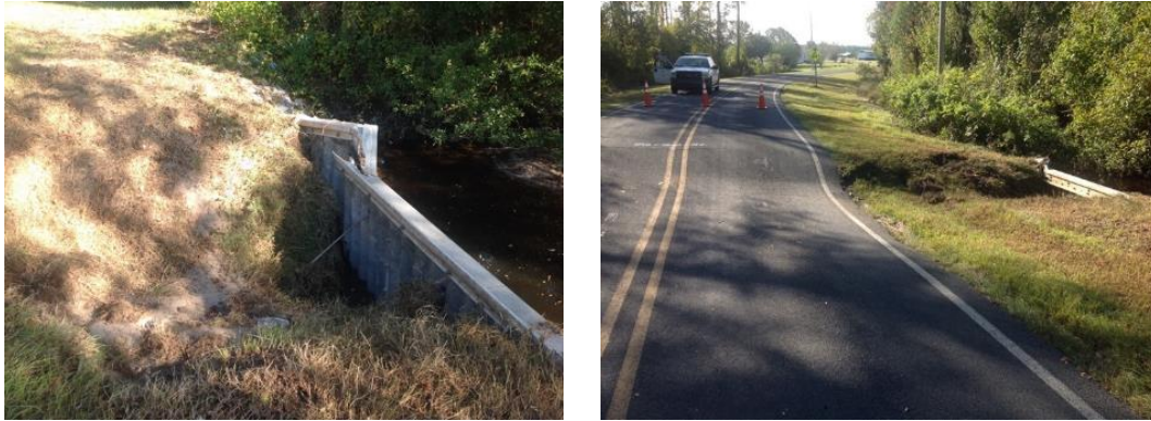
Figure 23. Photos of damage after Hurricane Matthew in Site 77-10-M.
