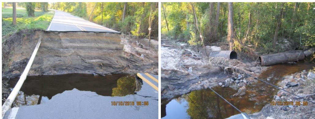
Figure 16. Photos of damage after Hurricane Matthew in Site 53-6-M.
