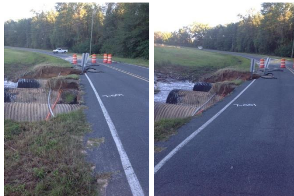
Figure 21. Photos of damage after Hurricane Matthew in Site 42-1-MF.
