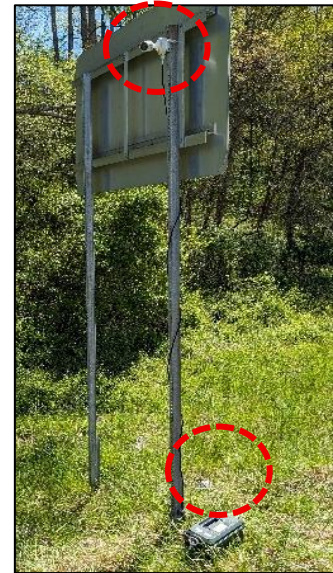
Figure 11. Example camera installation
