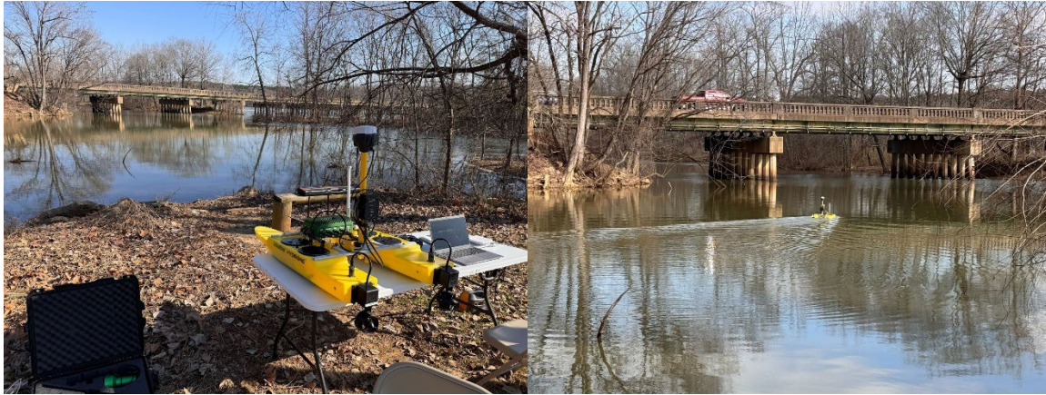
Figure 87: Left: Setup location prior to deployment near the west side of the bridge. Right: HyDrone transiting towards survey area (Bent 1 and 2 in view).
