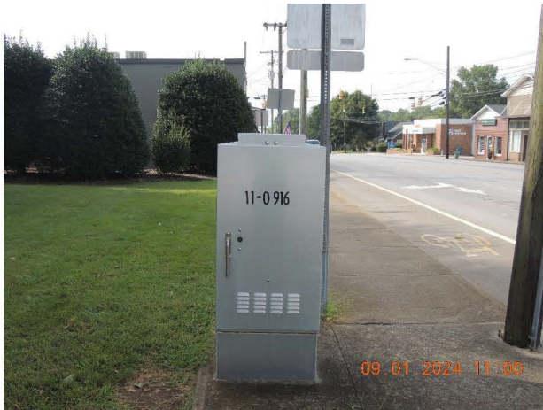
Intersection Signal Box
