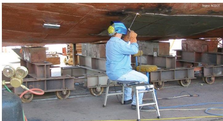
Image Caption: A boat welder works on a steel hull plate for an NCDOT ferry vessel.
