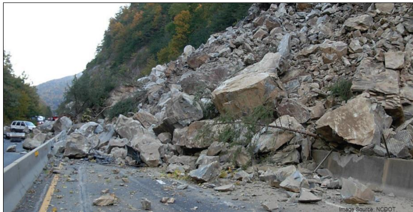
Figure 1. Rockslide on Interstate I-40
