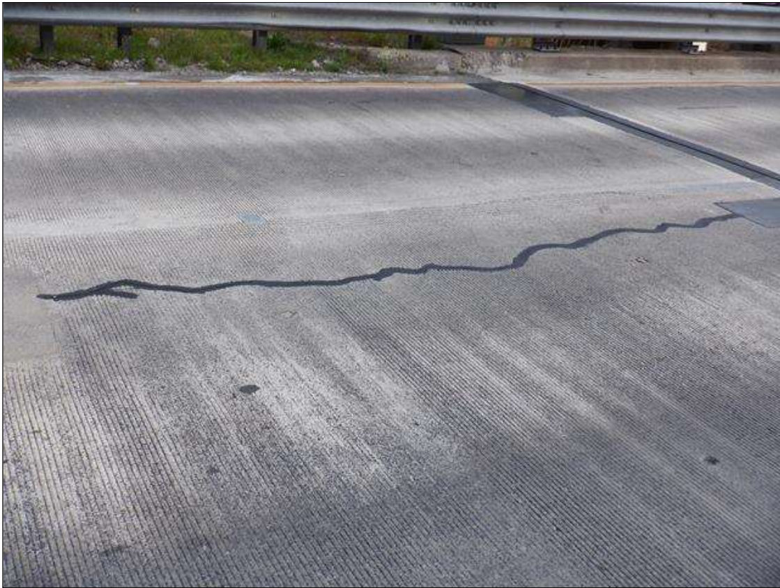
Approach 1 : 15 FEET SEALED LONGITUDINAL CRACK NEAR CENTERLINE
