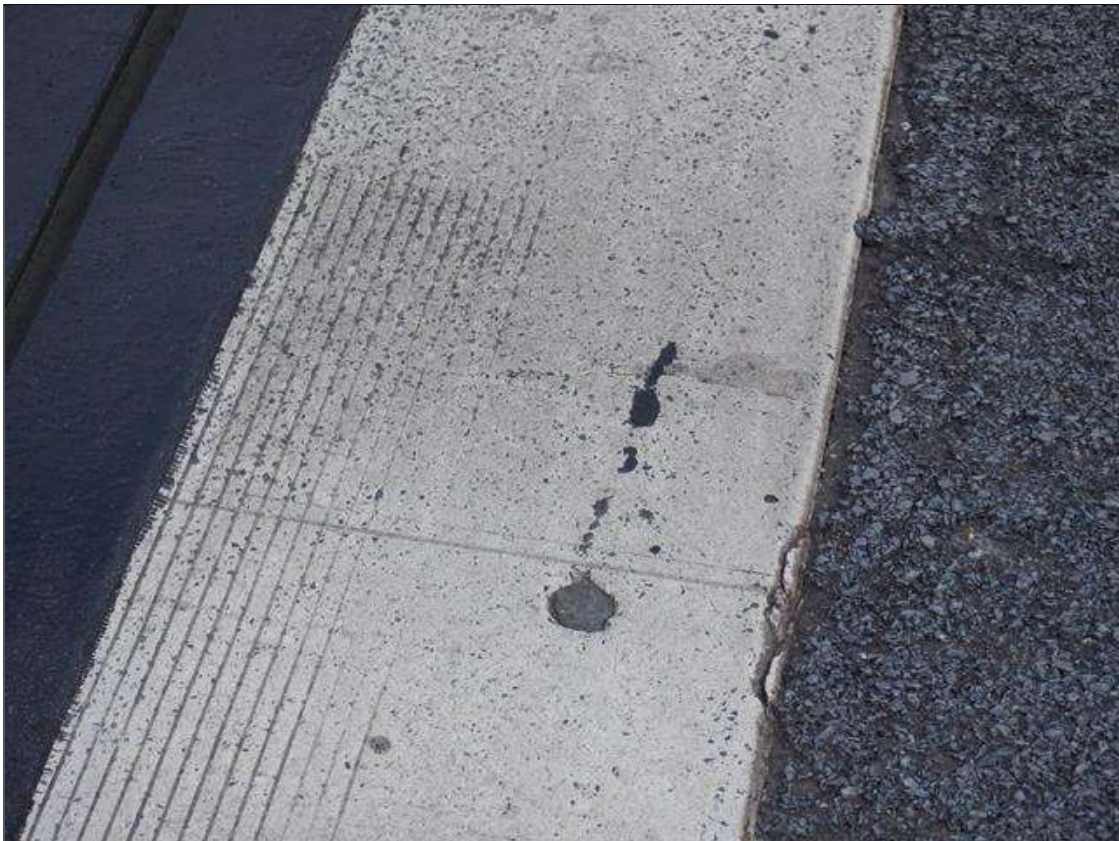
Approach 2 : 18 INCHES X UP TO 1/4 INCHES LONGITUDINAL CRACK IN EAST LANE
