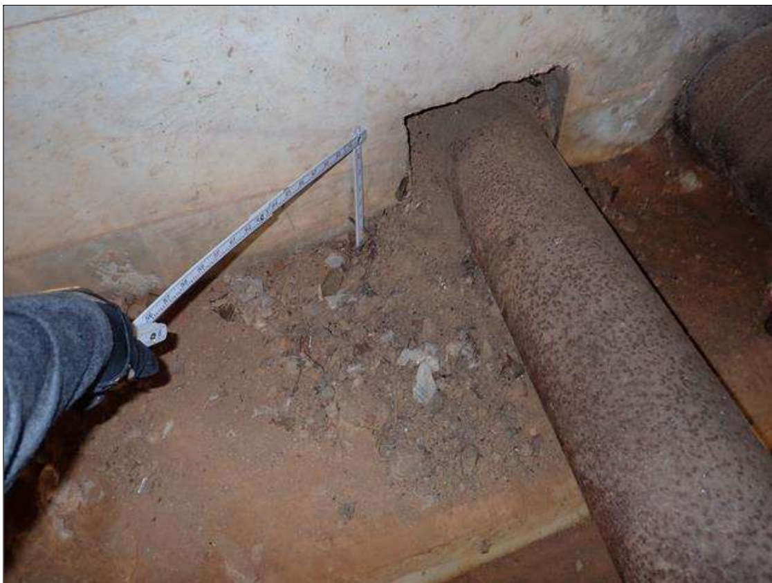
End Bent 2 Abutment: (PAR) SOIL INFILTRATION THROUGH UTILITY ACCESS HOLE, BAY 9.
