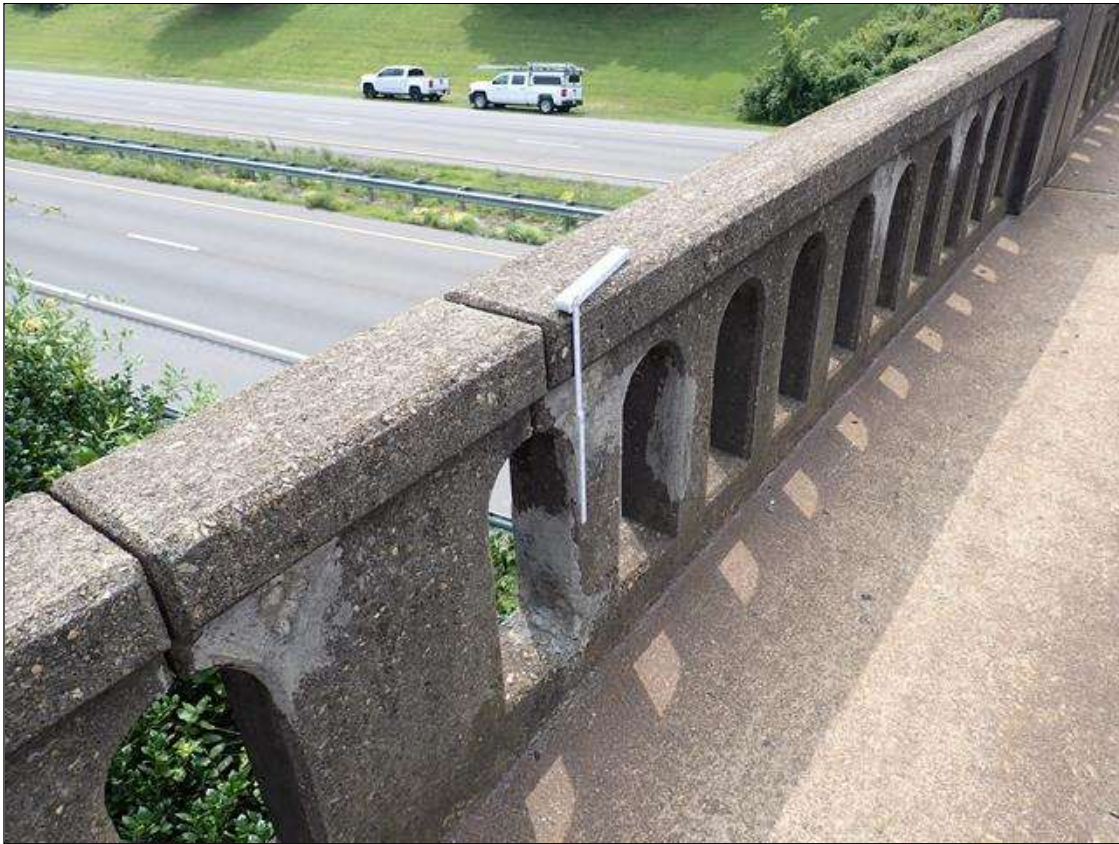
Span 4 Right Bridge Rail: SPAN 4 RIGHT RAIL HAS (7) PATCHED AREAS (UP TO 1 FOOT X 8 INCH) WITH HAIRLINE CRACKS.
