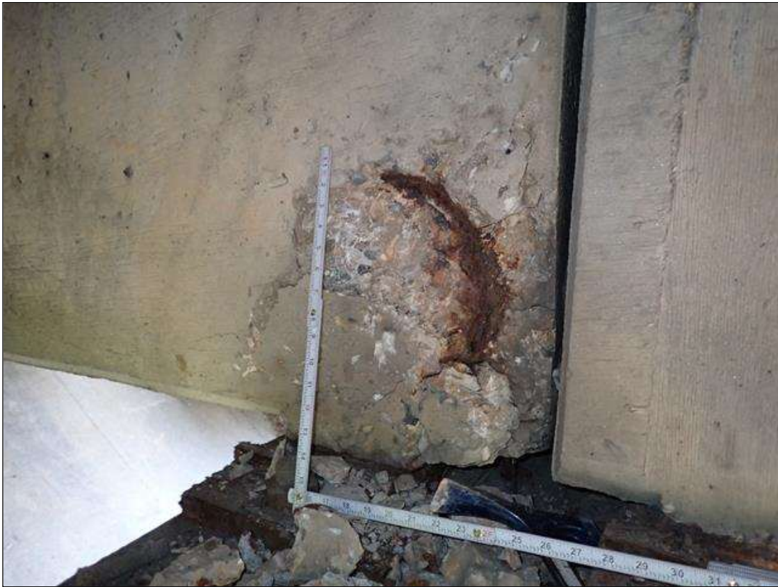
Span 4 Beam 8: (PAR) at bent 3, west face, spall/delamination (17 inch x 15 inch x 1.5 inch deep) with exposed rusted rebar (approximately 25 percent loss)
