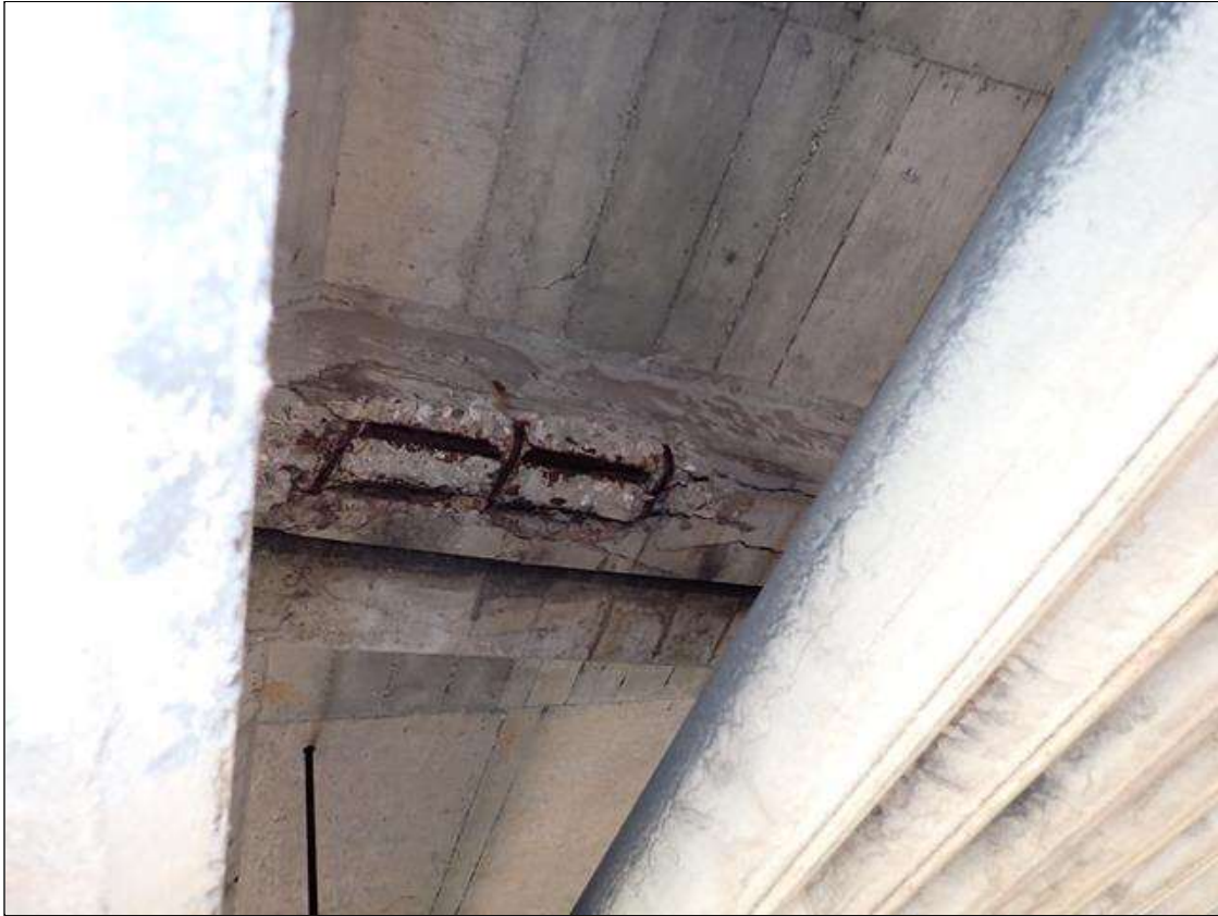
Span 3 Beam 8: (PAR) at bent 2, bay 8 end diaphragm, spall/delamination (full length x full width x 8 x 2 inch deep) with exposed rusted rebar (approximately 25 percent loss)
