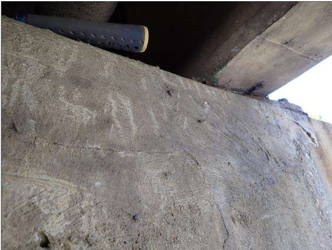
Bent 3 Cap 1: (PAR) BENT 3 CAP TOP AND SOUTH FACE BAY 9. HAS AN UNSOUND PATCHED AREA 6 FOOT X INCH X 12 INCH WITH SCATTERED HAIRLINE CRACKS, EFFLORESCENCE AND RUST STAINS
