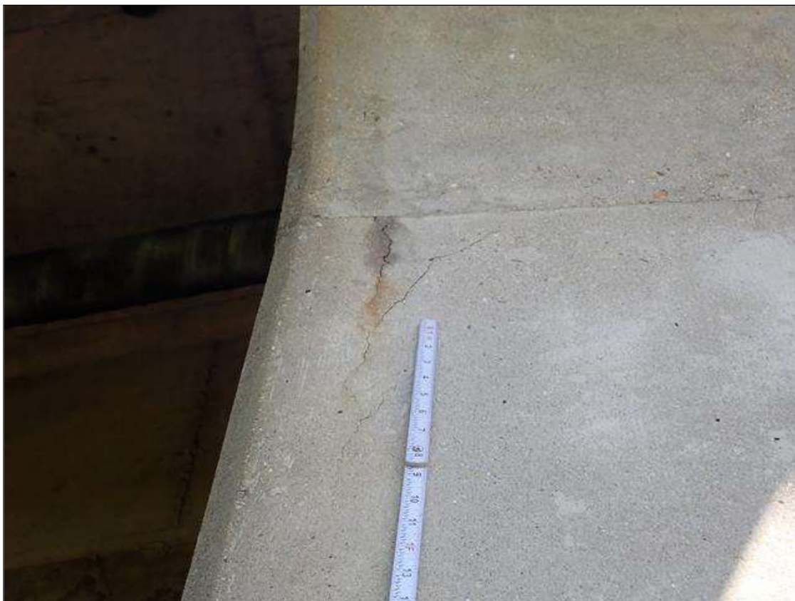
Bent 3 Pile 1: (PAR) MULTIPLE UP TO 3 FOOT X 1/16 INCH VERTICAL CRACKS WITH RUST STAINING, AT RANDOM THROUGHOUT.
