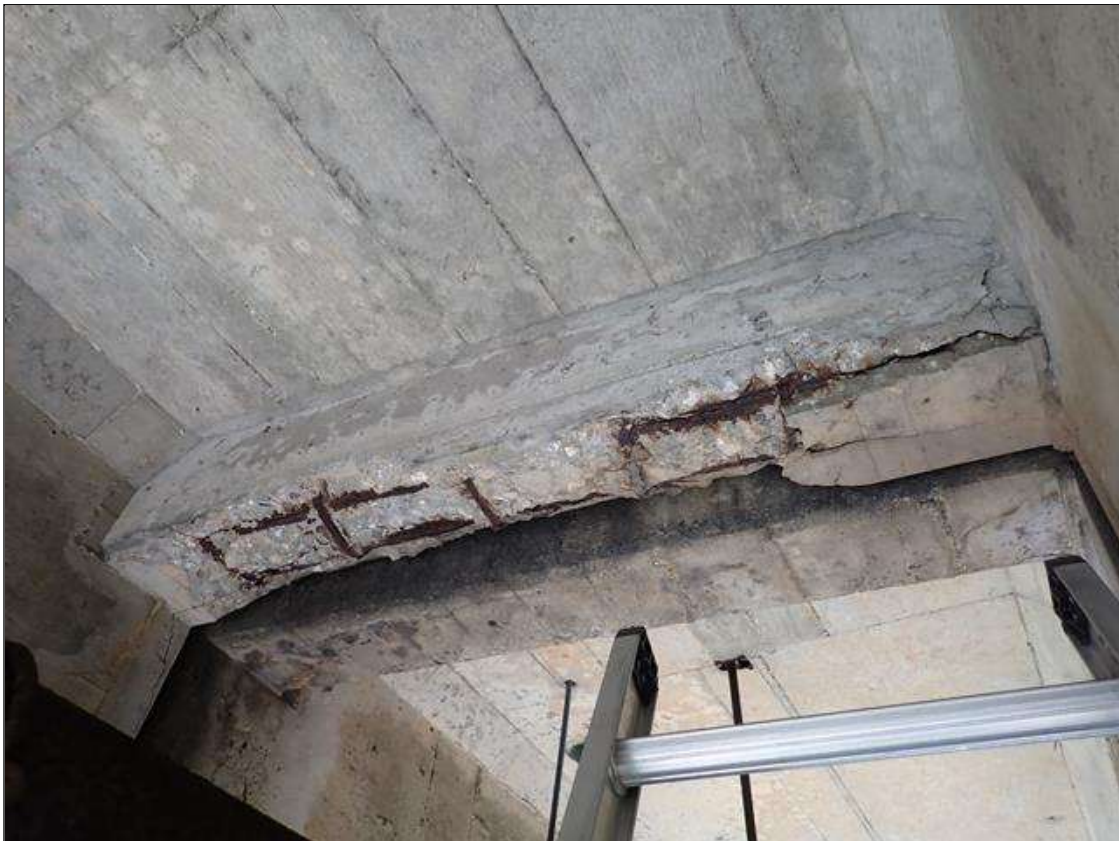
Span 3 Beam 9: (PAR) 6 FOOT X 1 FOOT X 8 INCH X 2 INCH DEEP SPALL WITH EXPOSED REINFORCING WITH APPROXIMATELY 25 PERCENT LOSS, IN BENT 2 DIAPHRAGM, BAY 9.
