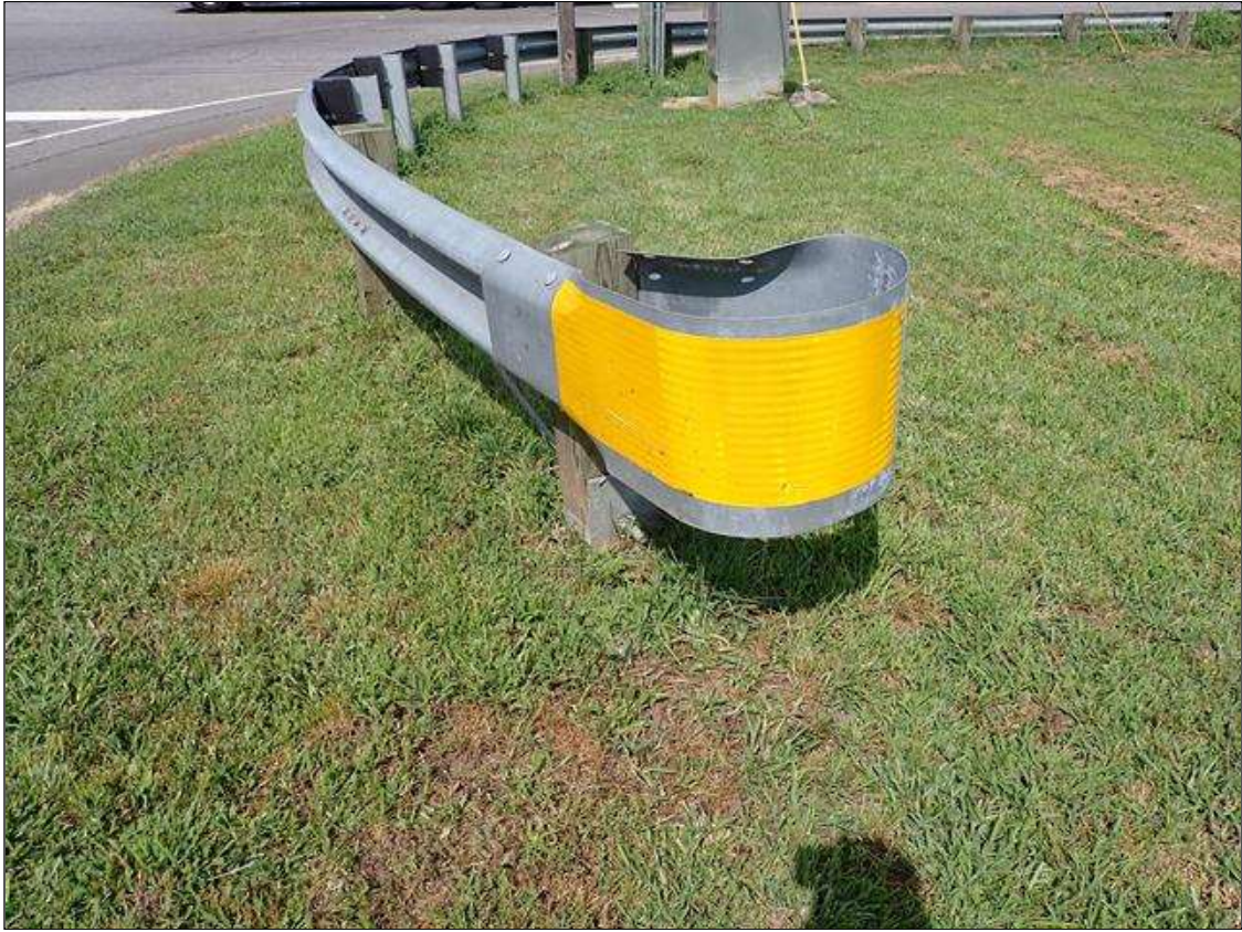
southeast guardrail termination
