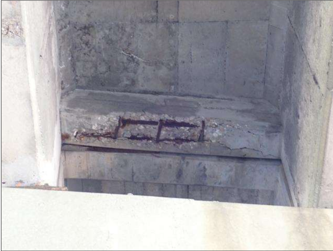
Span 2 Beam 3: (PAR) FULL LENGTH X FULL WIDTH X 4 INCH X 2 INCH DEEP SPALL/DELAMINATION WITH EXPOSED RUSTED REBAR WITH APPROXIMATELY 25 PERCENT LOSS IN BAY 3 DIAPHRAGM AT BENT 2.
