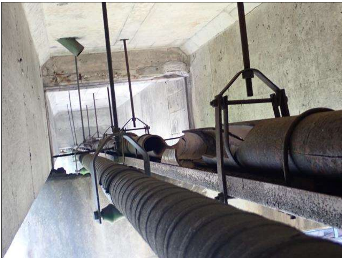
(PAR) span 4, bay 9 utility, near half, broken/cracked
