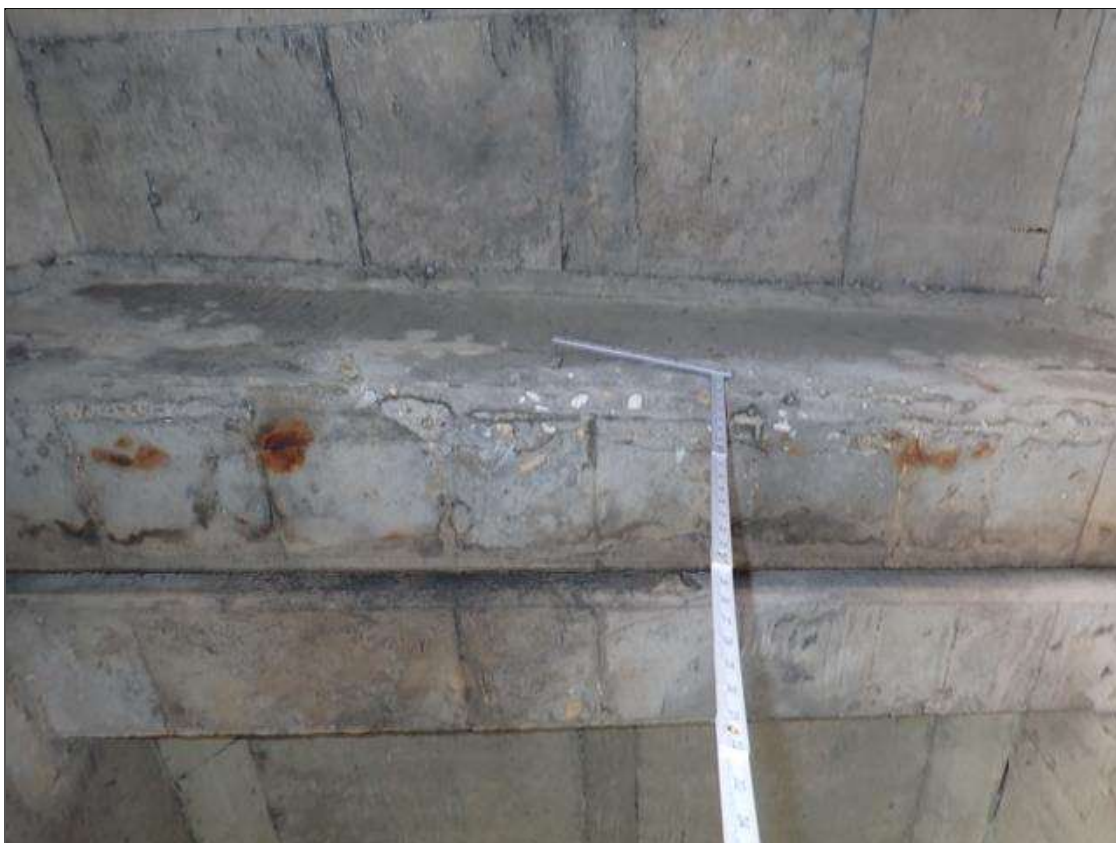
Span 3 Beam 3: (PAR) at bent 3, bay 3 end diaphragm, delamination (full width x 8 inch) with cracks (up to 1/4 inch deep) with rust stains
