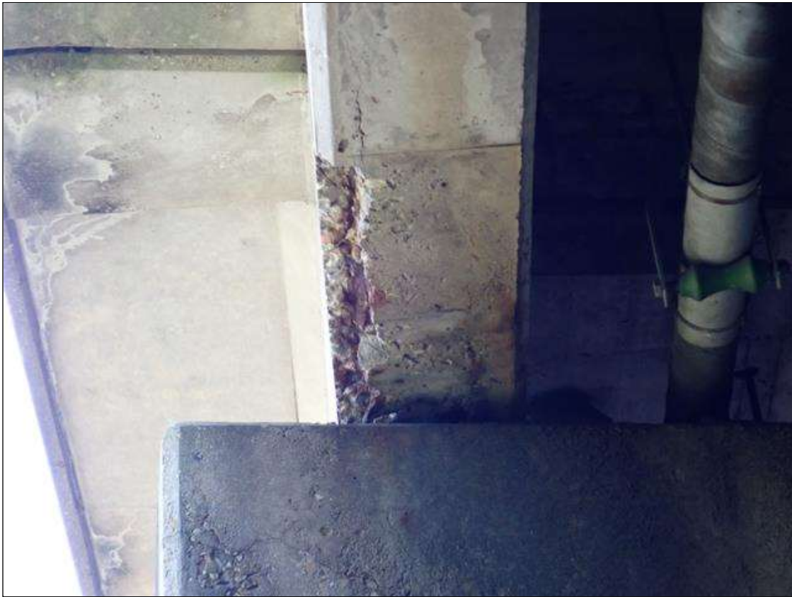
Span 4 Beam 10: (PAR) 2.5 FOOT X 2.5 INCH X 2 INCH DEEP SPALL/DELAMINATION WITH EXPOSED REBAR [SECTION LOSS UP TO 1/16 INCH DEEP], EAST AND BOTTOM FACES, AT BENT 3.
