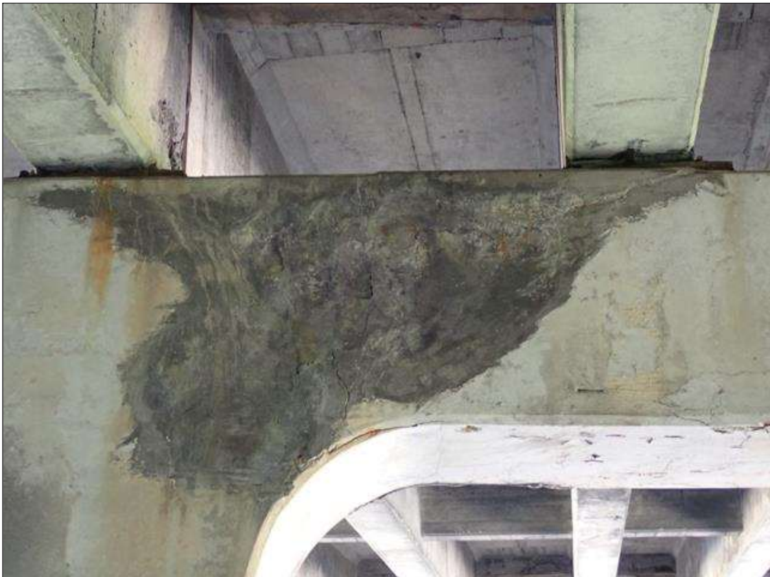
Bent 3 Cap 1: (PAR) BENT 3 CAP NORTH FACE BAY 6. FAILED PATCH [7 FOOT X UP TO 40 INCH] WITH MULTIPLE ADJACENT DELAMINATION [UP TO 28 INCH X 18 INCH], RUST STAIN AND EFFLORESCENCE
