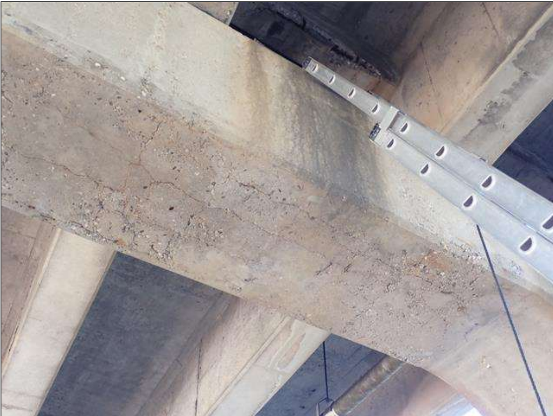
Bent 2 Cap 1: (PAR) 8 FOOT X 3 FOOT DELAMINATION WITH MAP CRACKING UP TO 1/16 INCH WITH RUST STAINS, BOTTOM FACE, BETWEEN PILES 1 AND 2.
