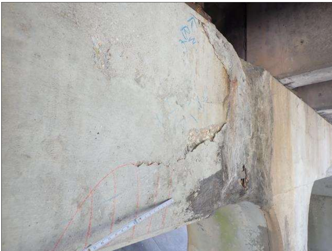
Bent 3 Cap 1: (PAR) south face in bay 6, failed patch (5 foot x full height x 3 inch deep) with exposed rusted rebar (approximately 25 percent loss)
