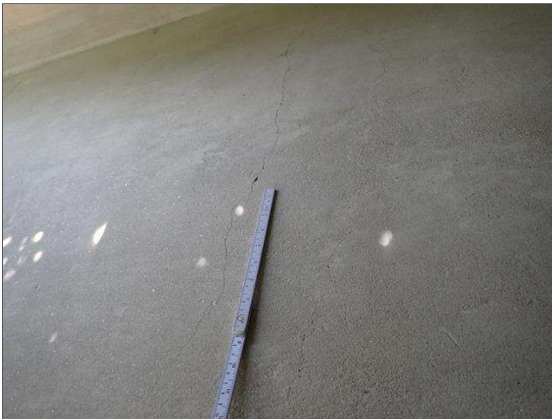
Span 4 Beam 10: along the length of the beam, vertical cracks (up to 1/32 inch x full height) at random
