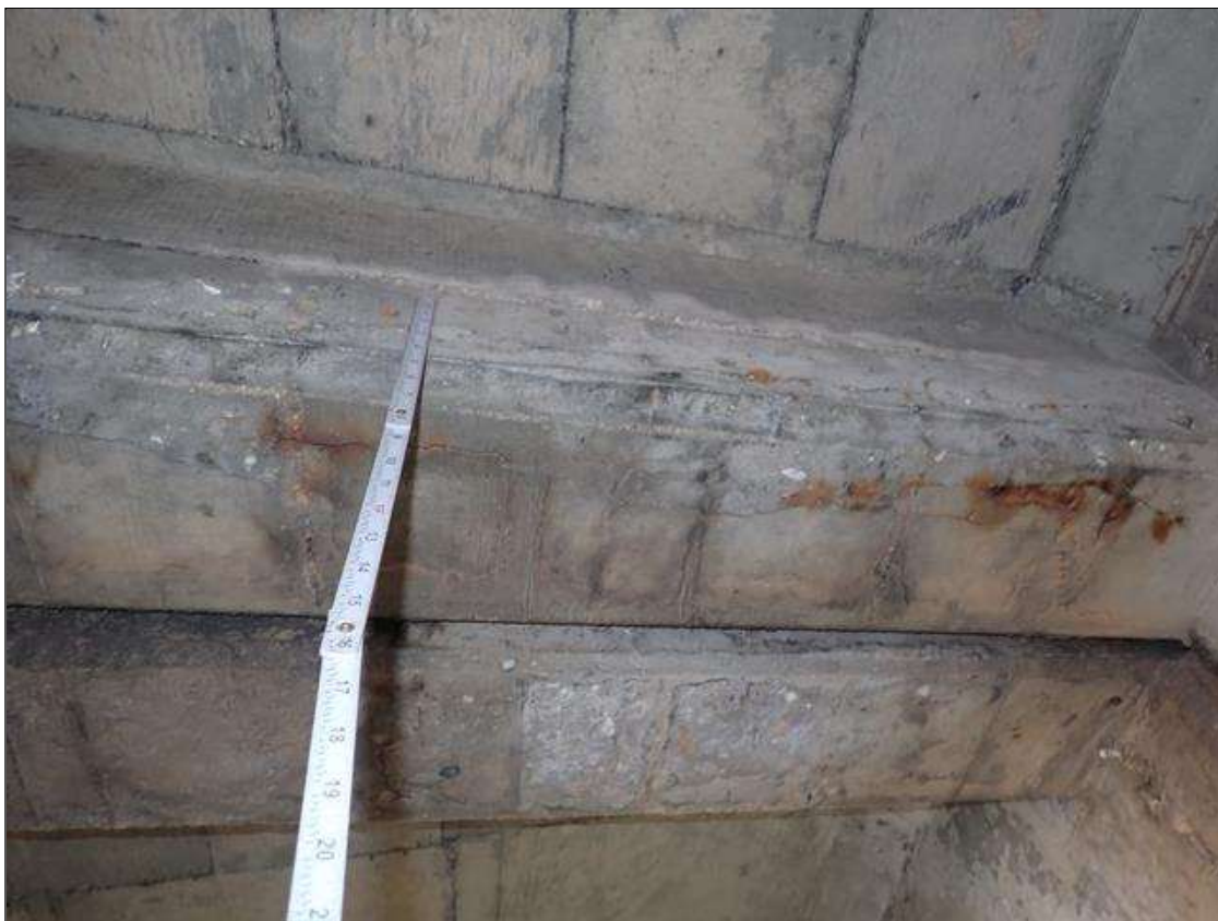
Span 3 Beam 4: (PAR) at bent 3, bay 4 end diaphragm, delamination (full width x 5 inch) with cracks (up to 1/4 inch deep) with rust stains
