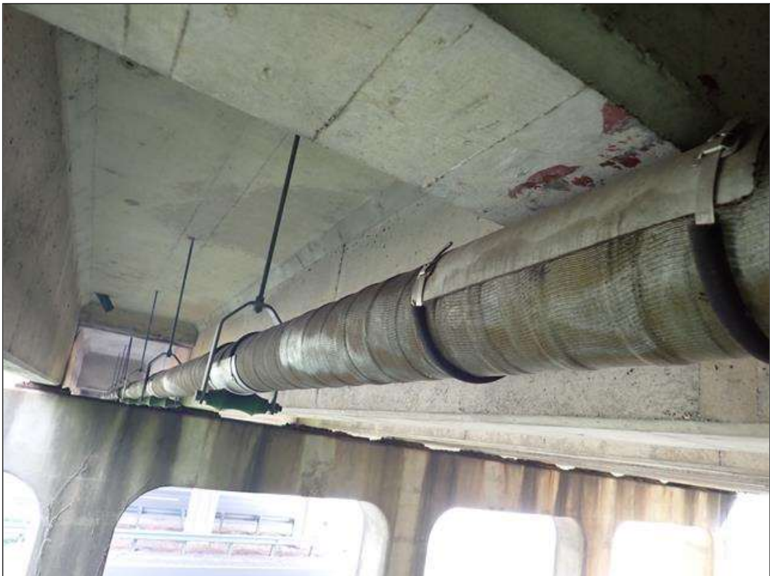
bay 1, gas line (6 inch diameter)
