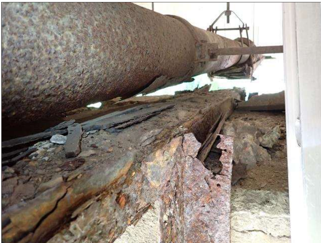
(PAR) at bent 2, bay 9 utility, metal platform, corroded and sheared
