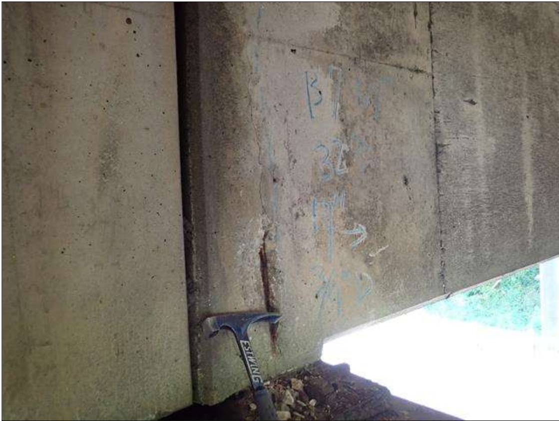
Span 2 Beam 7: (PAR) SPAN 2 BEAM 7 WEST WEB OVER BENT 2. HAS A CRACK/SPALL AND DELAMINATED AREA WITH REBAR EXPOSED. AREA IS: 7 INCH X 32 INCH X 3/4 INCH DEEP. WITH EXPOSED RUSTED REINFORCING WITH APPROXIMATELY 25 PERCENT LOSS
