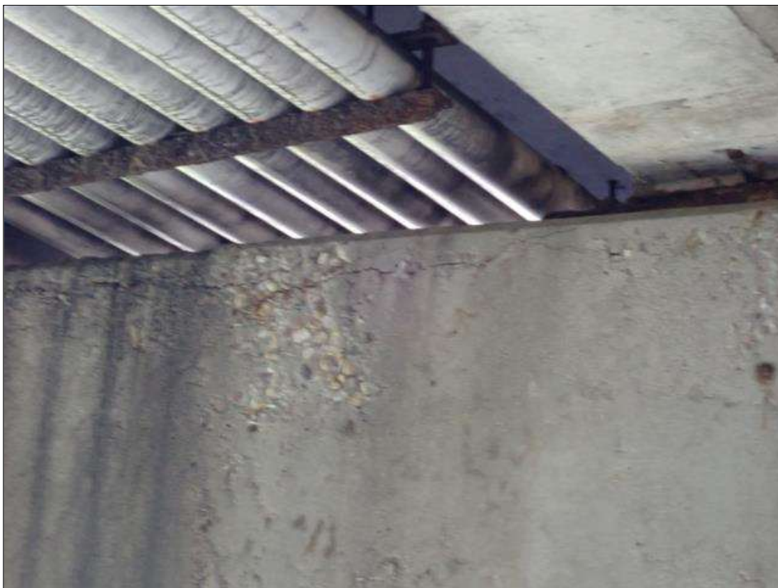
Bent 3 Cap 1: along the length of the cap, near top, longitudinal cracks (up to 1/8 inch x 8 foot) at random
