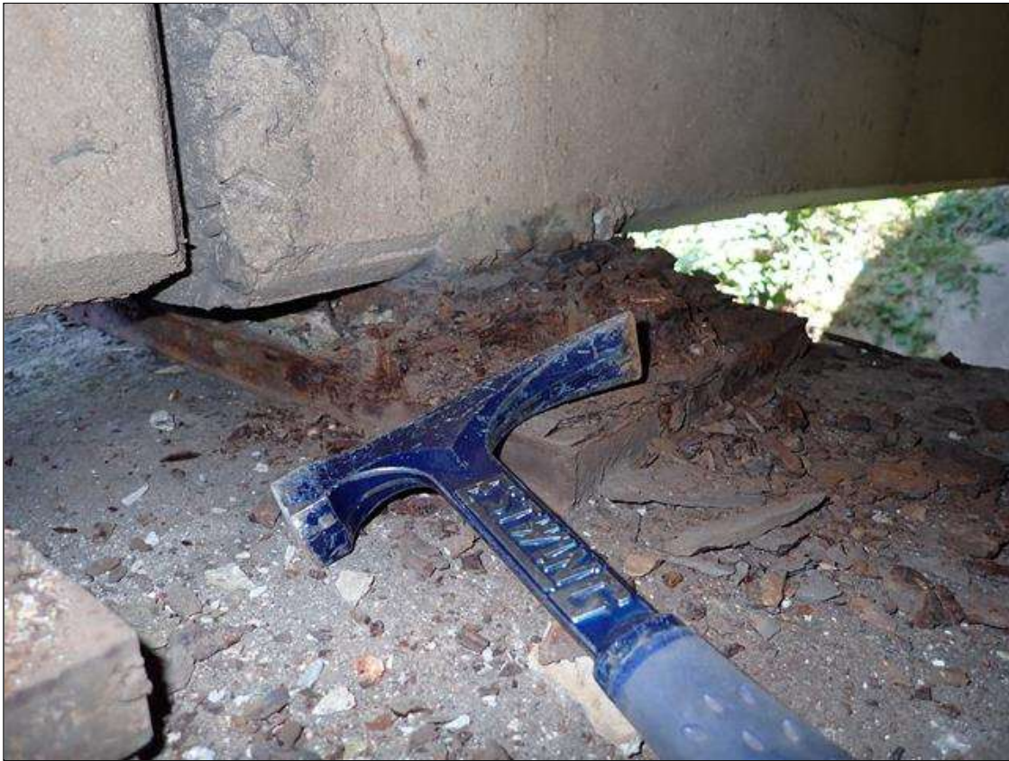
Span 4 Beam 1 - Near Bearing 1: active corrosion with section loss [up to 1/8 inch loss on plates]; anchor bolts, corrosion with section loss [approximately 75 percent remaining]
