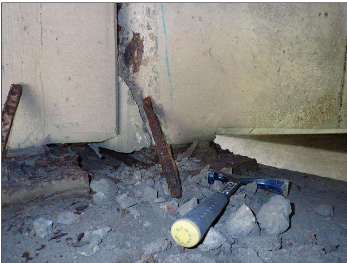
Span 4 Beam 6 - Near Bearing 6: (PAR) active corrosion with section loss [up to 1/16 inch loss on plates]; east guide rail, sheared
