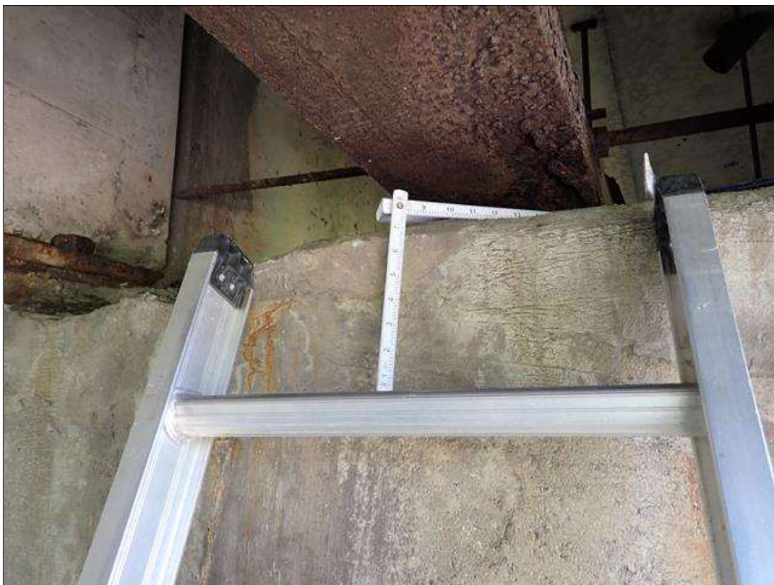
Bent 3 Cap 1: (PAR) BENT 3 CAP TOP AND SOUTH FACE BAY 9. HAS AN UNSOUND PATCHED AREA 6 FOOT X INCH X 12 INCH WITH SCATTERED HAIRLINE CRACKS, EFFLORESCENCE AND RUST STAINS
