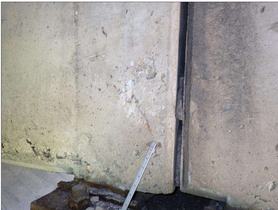
Span 4 Beam 4: at bent 3, west face, spall/delamination (10 inch x 6 inch x 1/2 inch deep)
