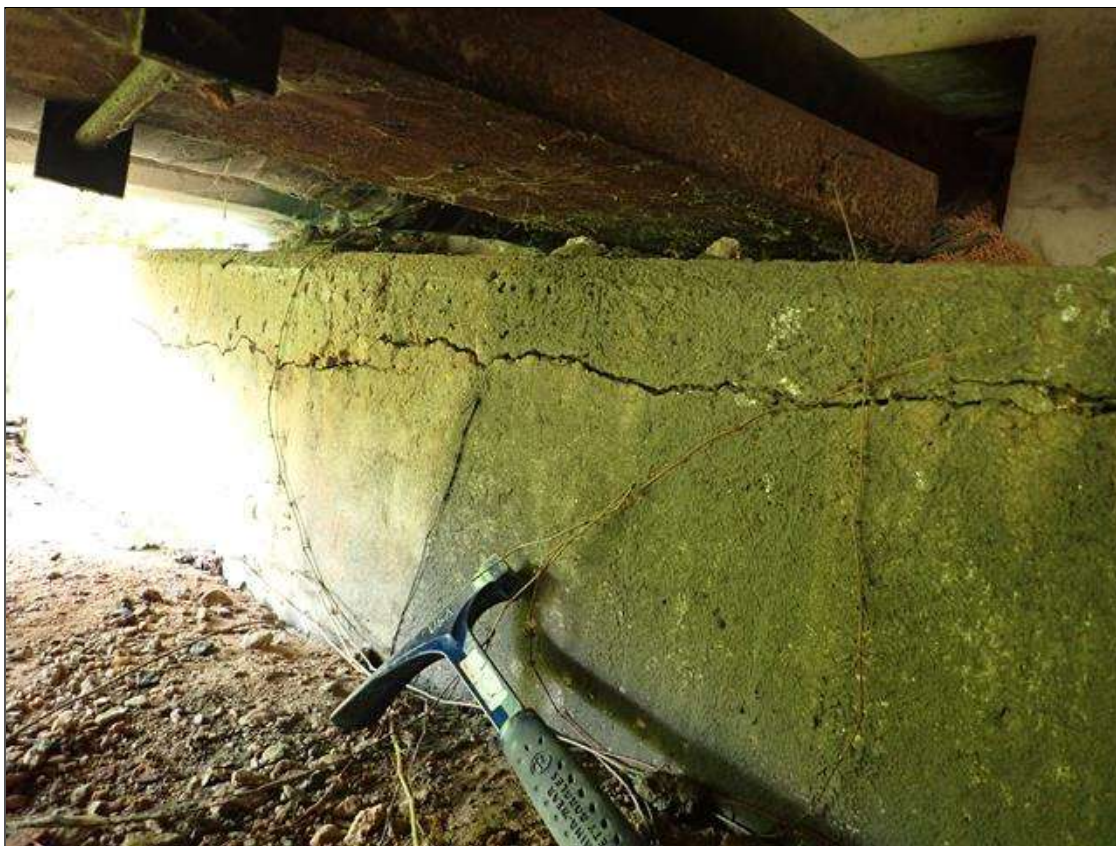
End Bent 1 Cap 1: (PAR) END BENT 1 CAP HAS A DELAMINATION 8 FOOT X 6 INCH X 6 INCH WITH CRACKS UP TO 1/4 INCH CRACKS WITH EFFLORESCENCE AND RUST STAINS VISIBLE, UNDER BAY 9.
