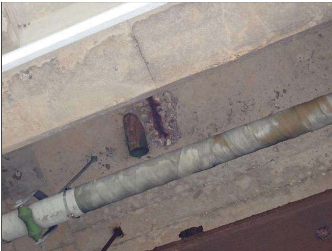
Span 2 Deck: (PAR) underside of deck in bay 9 near bent 1, (2) spalls (up to 18 inch x 1 foot x 1 inch deep) with exposed rusted rebar
