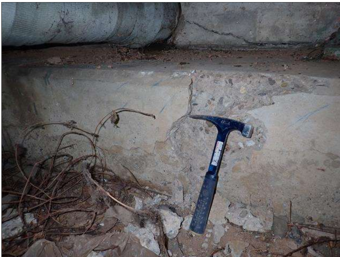
End Bent 2 Cap 1: below bay 1, spall/delamination (7 foot x 15 inch x 4 inch x 2 inch deep)
