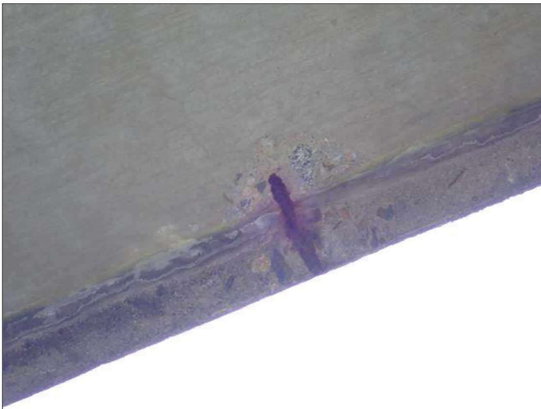
Span 4 Deck: (PAR) along underside left overhang, three [3] spalls [up to 6 inch diameter x 1/2 inch deep] with exposed rusted reinforcing [no loss noted]
