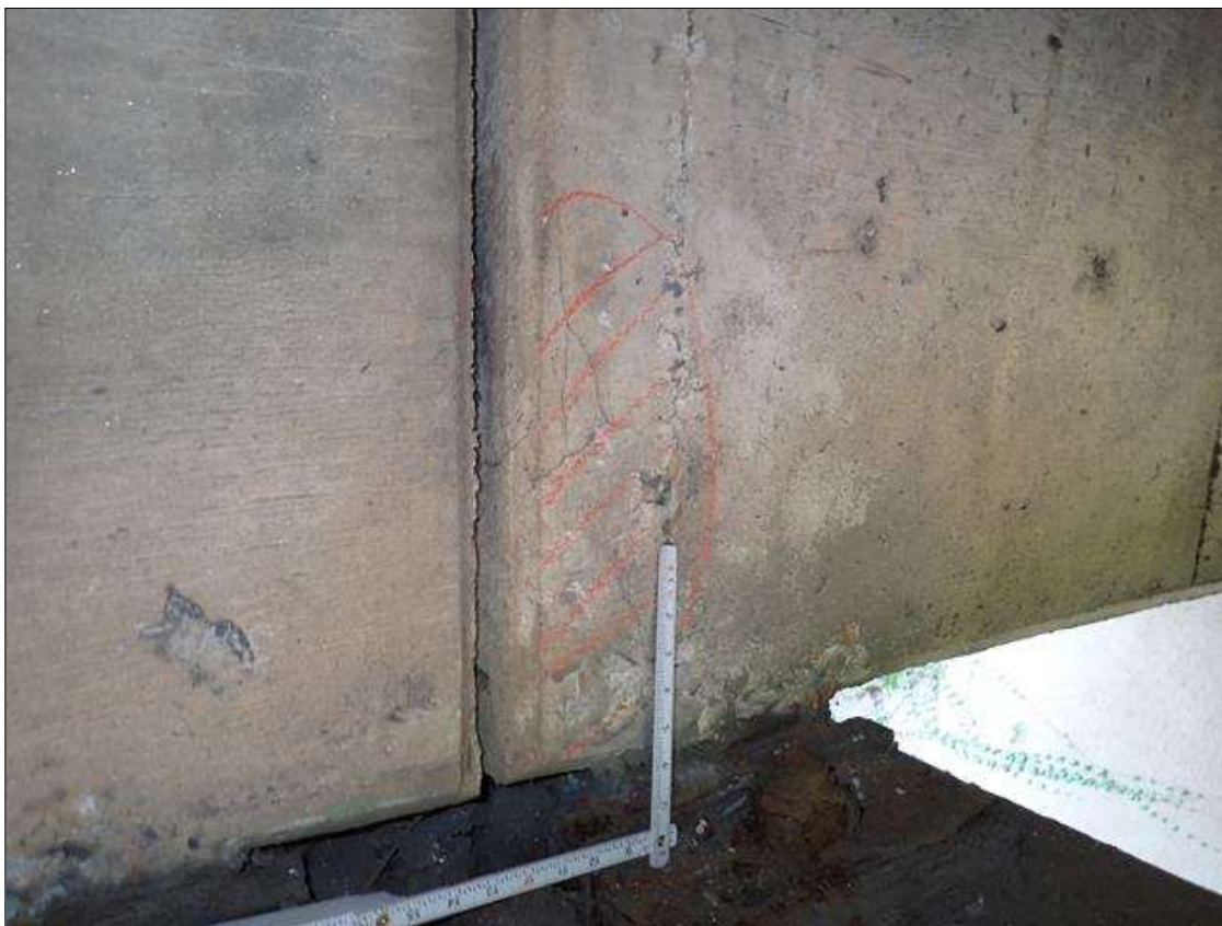
Span 4 Beam 3: at bent 3, east face, delamination (6 inch x 15 inch) with cracks (up to 1/32 inch)
