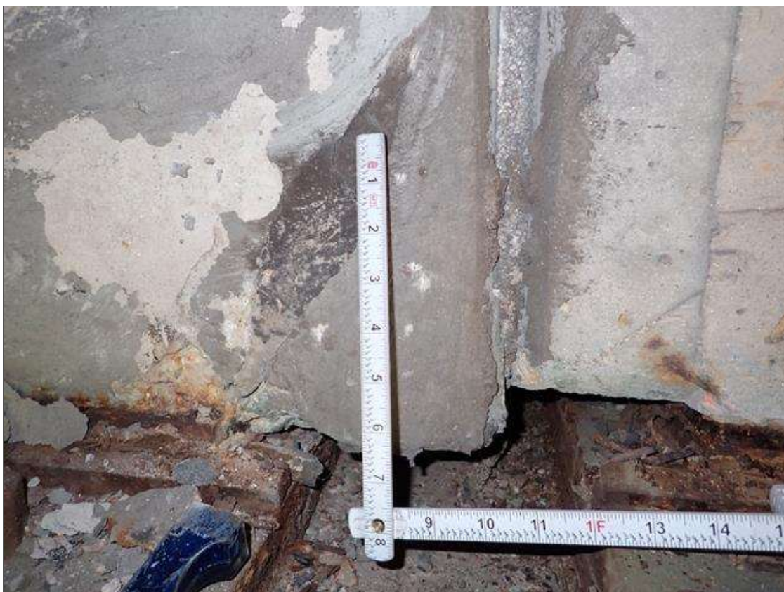
Span 4 Beam 6: at bent 3, west face, failed patch (8 inch x 8 inch x 3/4 inch deep)
