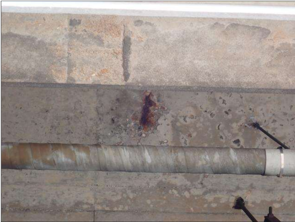
Span 2 Deck: (PAR) underside of deck in bay 9 near bent 1, (2) spalls (up to 18 inch x 1 foot x 1 inch deep) with exposed rusted rebar
