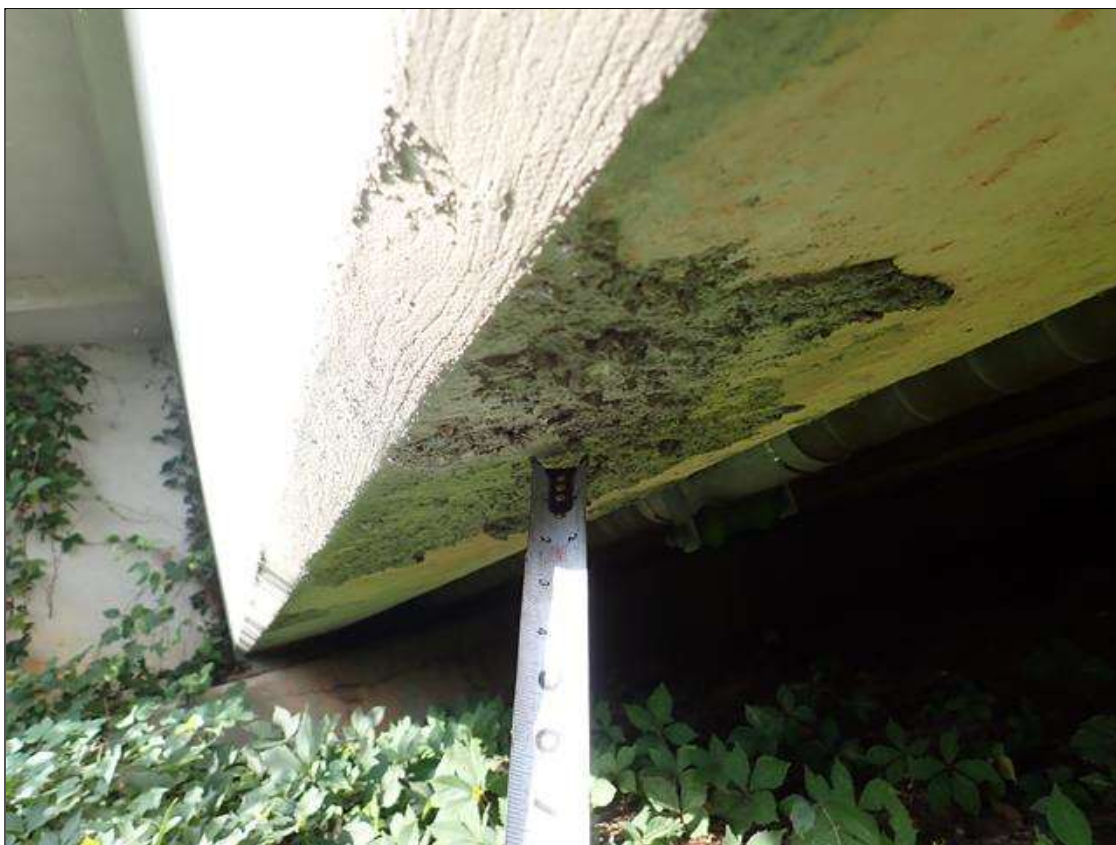
Span 1 Beam 10: 10.5 foot from end bent 1, underside, patched area (2 foot x 8 inch)
