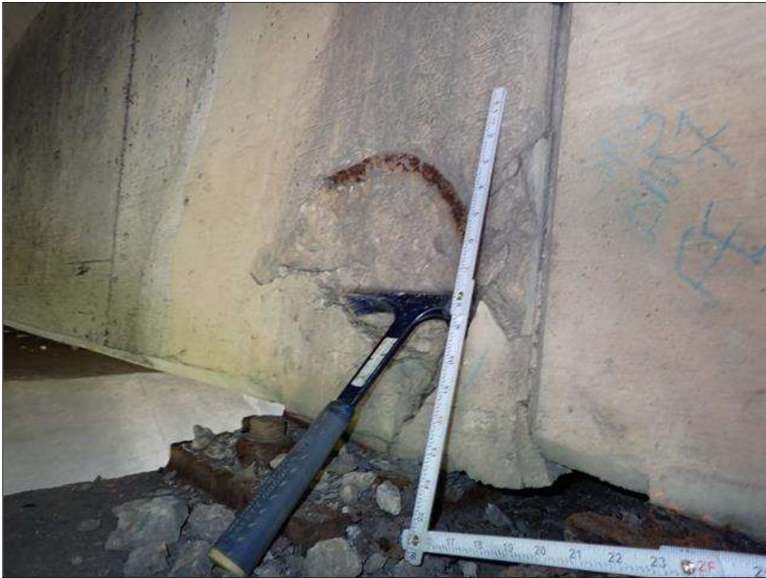
Span 4 Beam 7: (PAR) SPAN 4 BEAM 7 WEST WEB OVER BENT 3. HAS A CRACK/SPALL AND DELAMINATED AREA WITH REBAR EXPOSED WITH APPROXIMATELY 25 PERCENT LOSS. AREA IS: 20 INCH X 15 INCH X 2 INCH DEEP.
