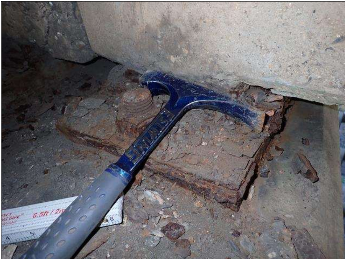
Span 2 Beam 5 - Near Bearing 5: active corrosion with section loss [up to 1/8 inch loss on plates]; anchor bolts, corrosion with section loss [approximately 75 percent remaining]
