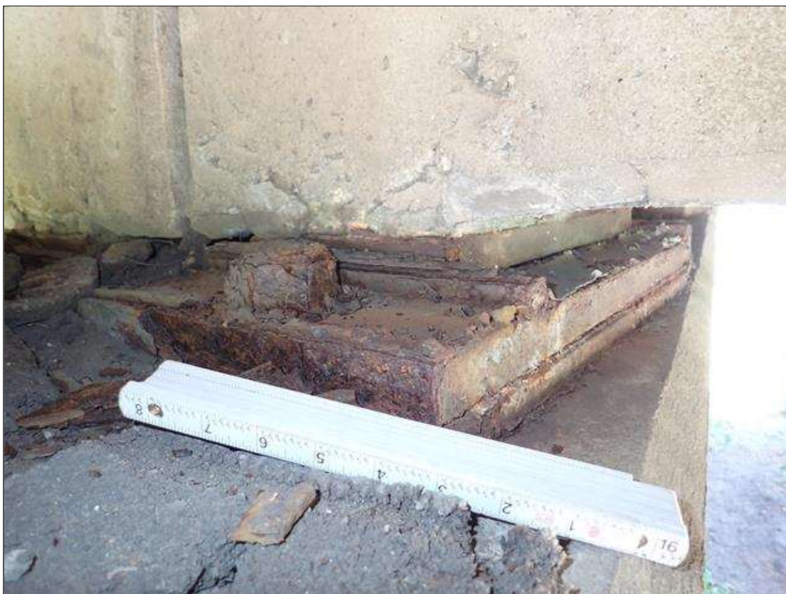
Span 3 Beam 3 - Far Bearing 3: active corrosion with section loss [up to 1/16 inch loss on plates]
