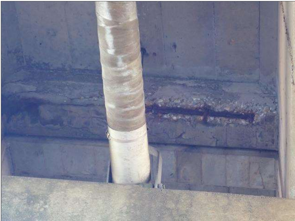
Span 2 Beam 1: (PAR) FULL LENGTH X FULL WIDTH X 4 INCH X 2 INCH DEEP SPALL WITH EXPOSED REINFORCING WITH APPROXIMATELY 25 PERCENT LOSS, IN BENT 2 DIAPHRAGM, BAY 1.
