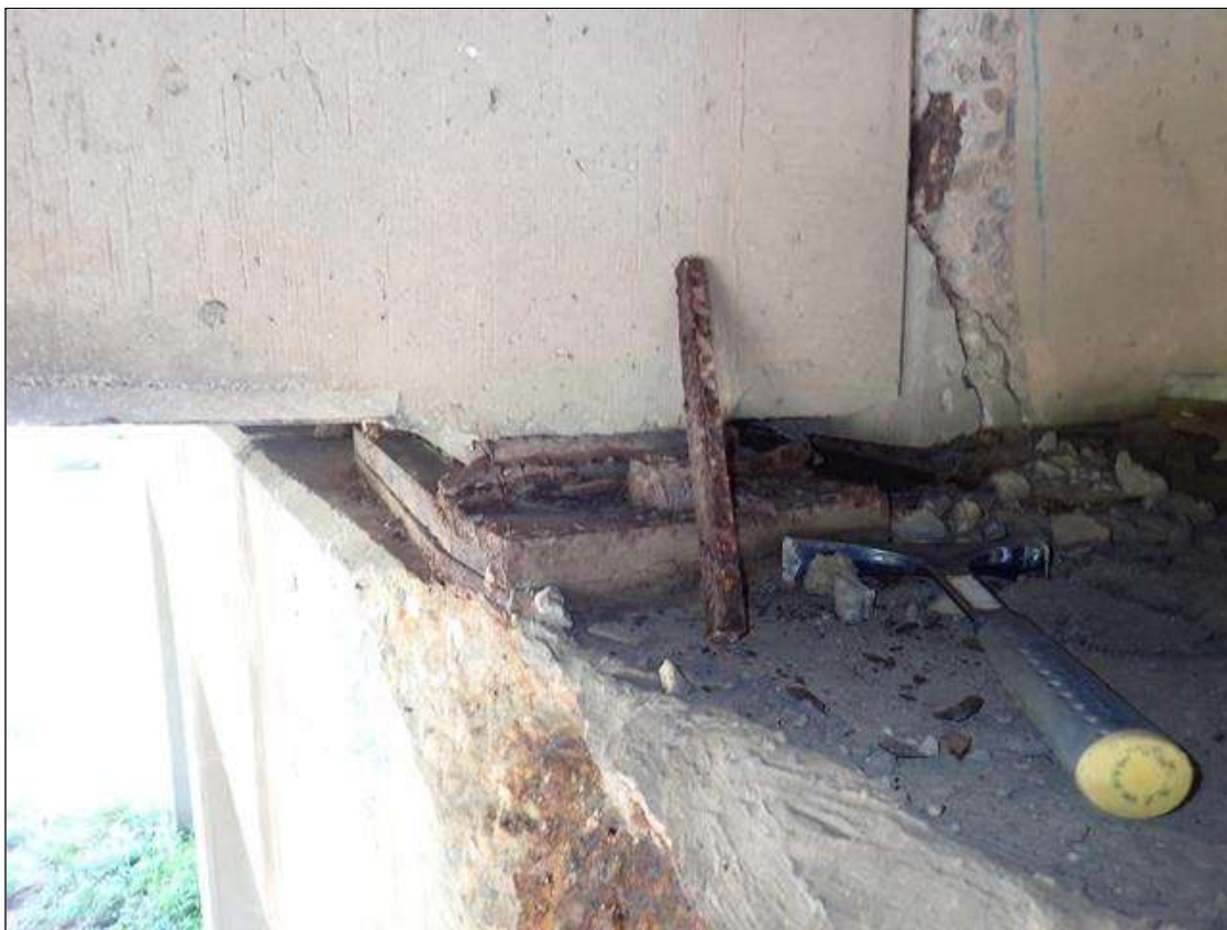
Span 3 Beam 6 - Far Bearing 6: (PAR) active corrosion with section loss [up to 1/16 inch loss on plates]; east guide rail, sheared
