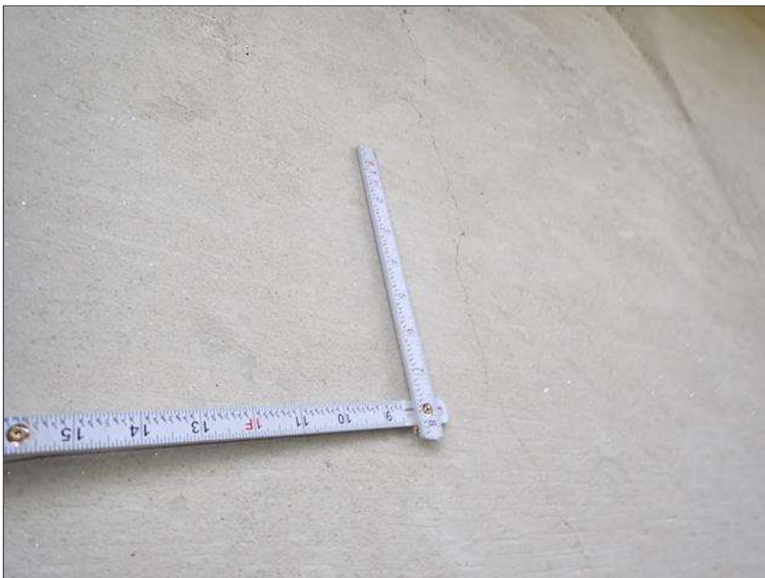
Span 4 Beam 1: along the length of the beam, vertical cracks (up to 1/32 inch x full height) at random
