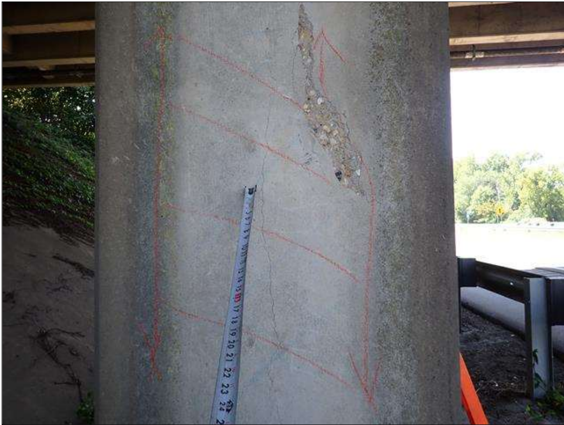
Bent 1 Pile 3: east and west faces, spall/delamination (21 inch x full height x 1/2 inch deep) with cracks (up to 1/32 inch)
