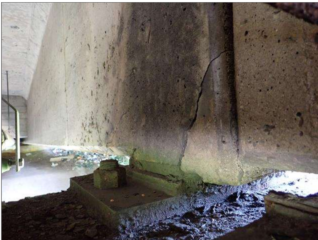
Span 4 Beam 10: West face at near end, delamination [3 foot x up to full height] with cracks [up to 1/8 inch]
