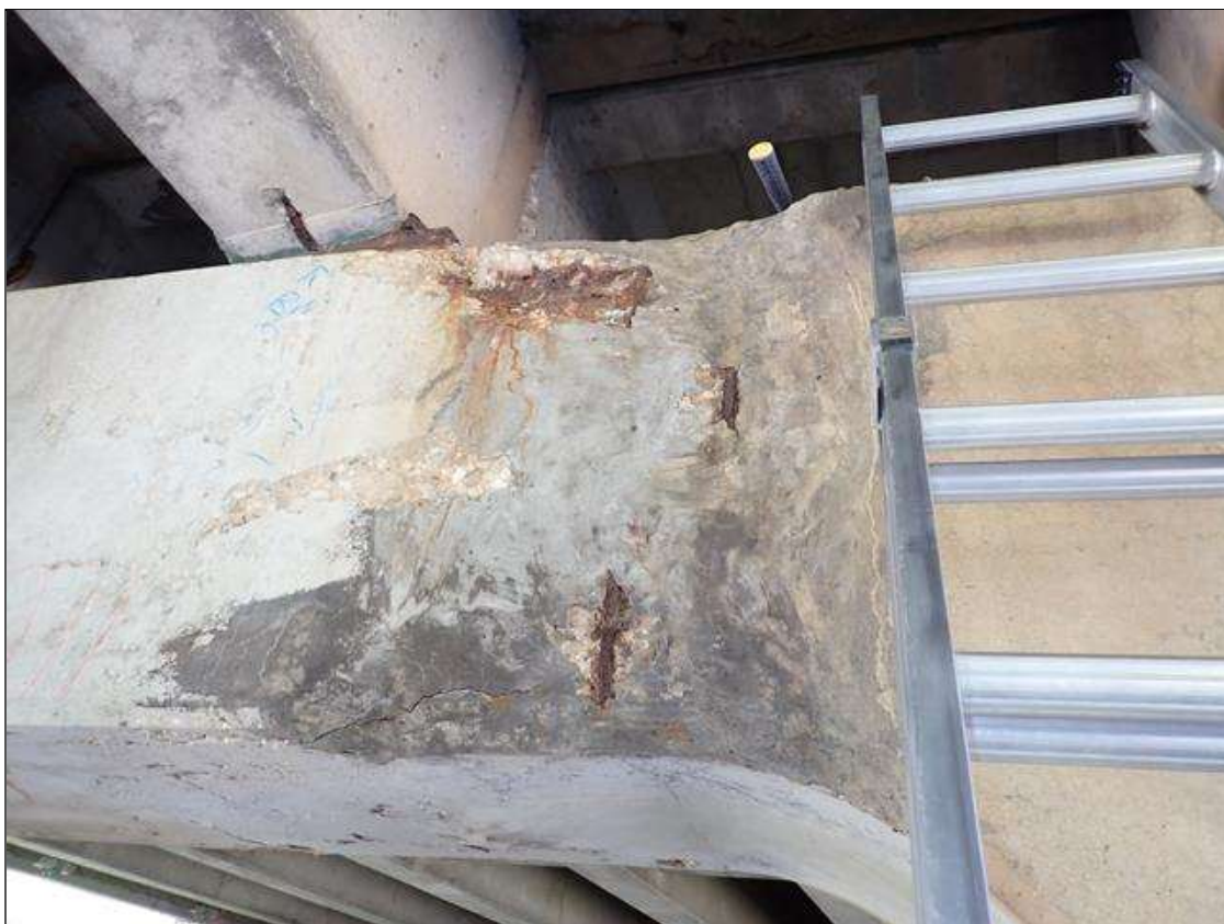
Bent 3 Cap 1: (PAR) south face in bay 6, failed patch (5 foot x full height x 3 inch deep) with exposed rusted rebar (approximately 25 percent loss)
