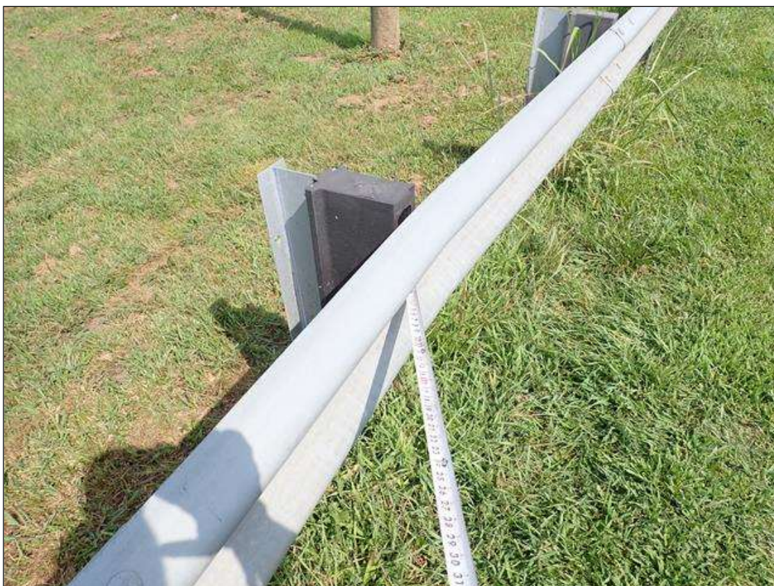
(PAR) northwest guardrail near termination, (2) areas of impact damage (up to 10 foot); 18 foot total
