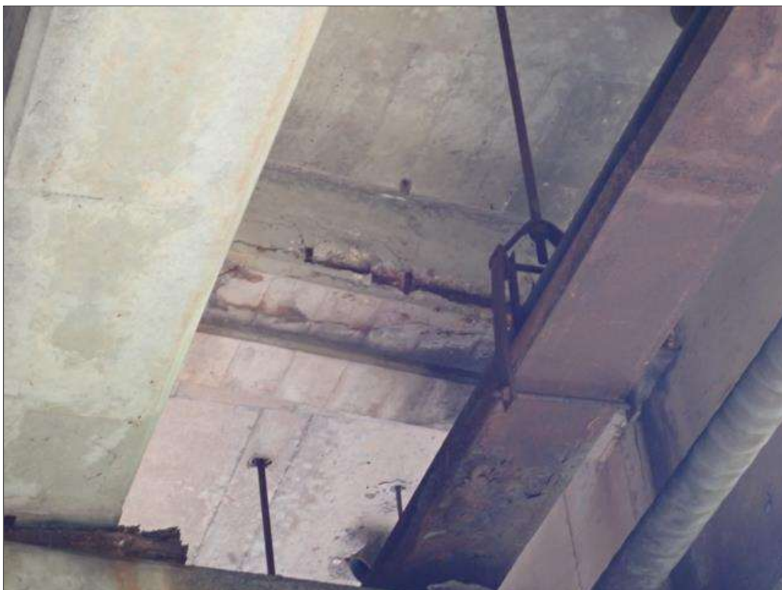
Span 1 Beam 9: (PAR) at bent 1, bay 9 end diaphragm, spall/delamination (full length x full width x up to full height x 1 inch deep) with exposed rusted rebar (approximately 25 percent loss)
