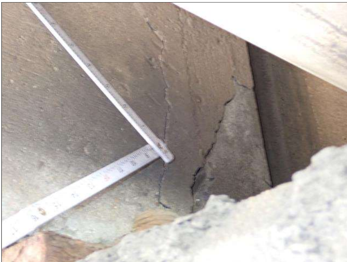
Span 2 Beam 9: at bent 1, west face, spall/delamination (8 inch x up to full height x 1 inch deep)
