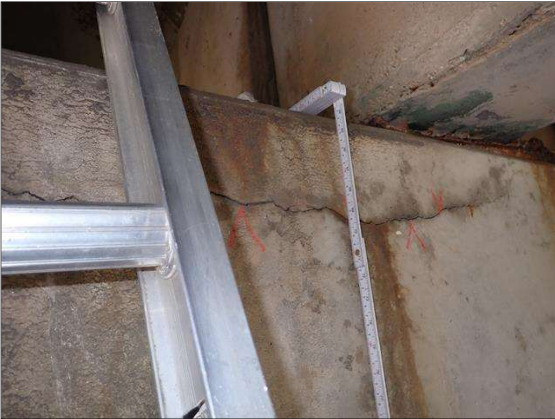
Bent 1 Cap 1: along the length of the cap, near top, longitudinal cracks (up to 1/16 inch x 8 foot) at random
