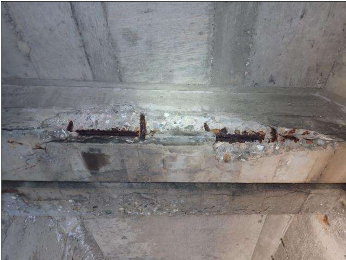
Span 3 Beam 2: (PAR) at bent 2, bay 2 end diaphragm, spall/delamination (full length x full width x 8 x 2 inch deep) with exposed rusted rebar (approximately 25 percent loss)
