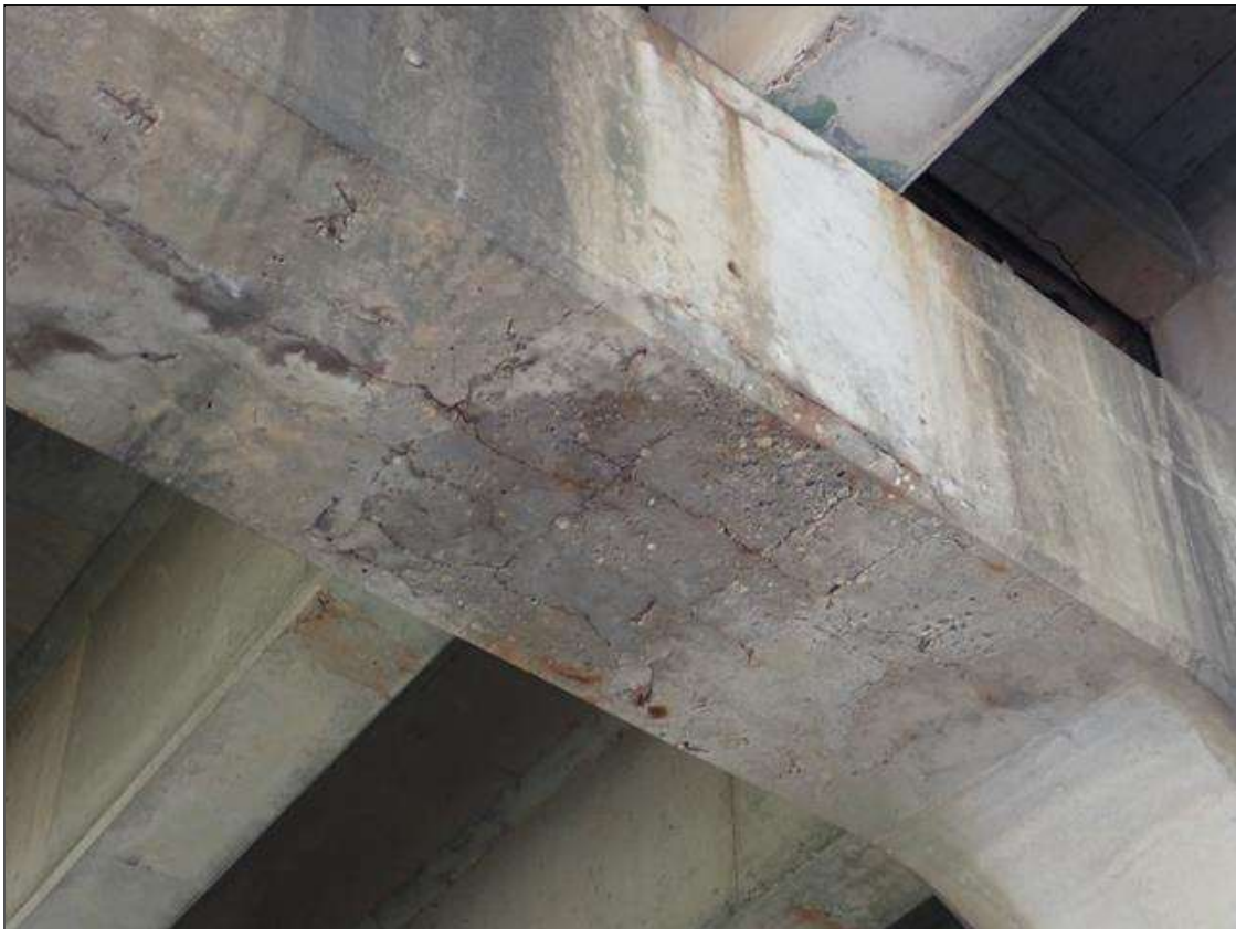
Bent 1 Cap 1: (PAR) underside of cap between columns, delaminations (up to 10 foot x full width) extending into vertical faces (up to 1 foot) with cracks (up to 1/8 inch) with rust stains
