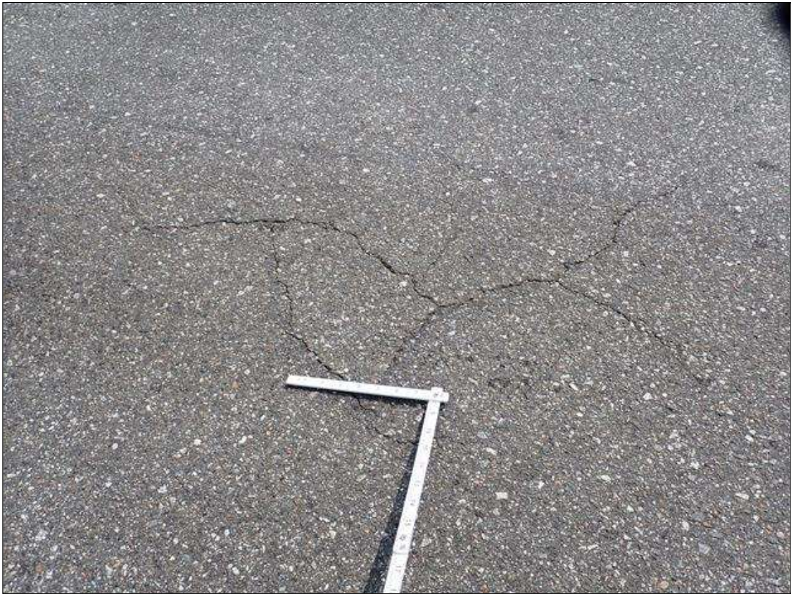
Span 2 Wearing Surface: throughout asphalt wearing surface, map cracks (up to 1/32 inch) at random
