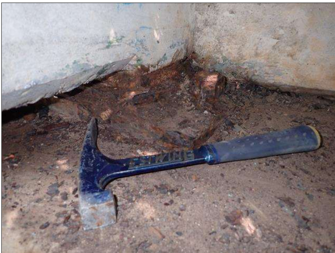
Span 4 Beam 10 - Far Bearing 10: active corrosion with section loss [up to 1/8 inch on plates]
