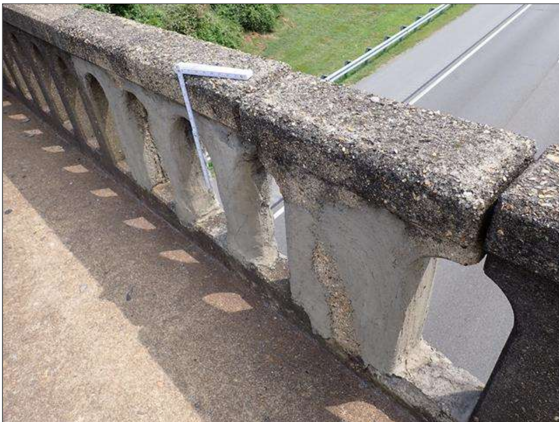
Span 3 Right Bridge Rail: SPAN 3 RIGHT RAIL HAS MULTIPLE PATCHED AREAS (2 FOOT X 7 INCH) WITH HAIRLINE CRACKS
