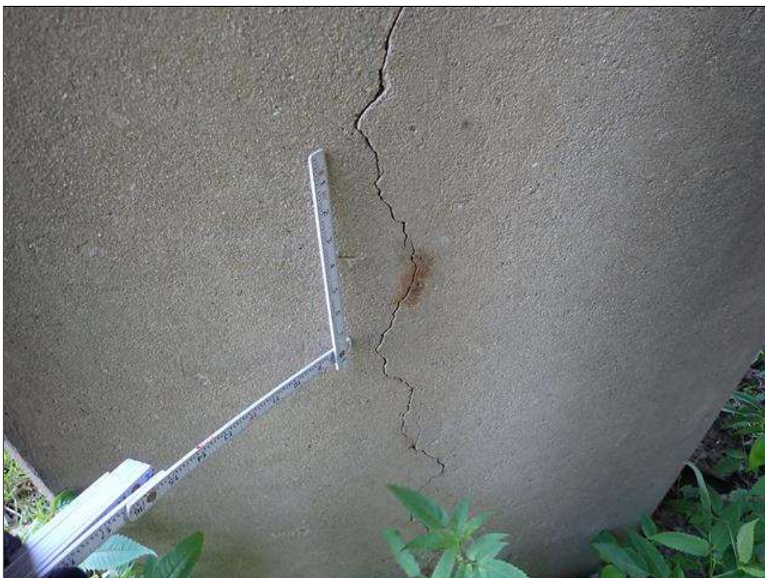
Bent 3 Pile 4: (PAR) MULTIPLE UP TO FULL HEIGHT X 1/16 INCH VERTICAL CRACKS WITH RUST STAINING, AT RANDOM THROUGHOUT.
