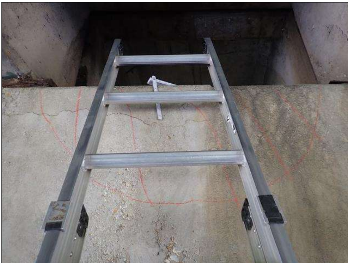
Bent 3 Cap 1: south face in bay 4, delamination (4 foot x 1.5 foot) with cracks (up to 1/32 inch)
