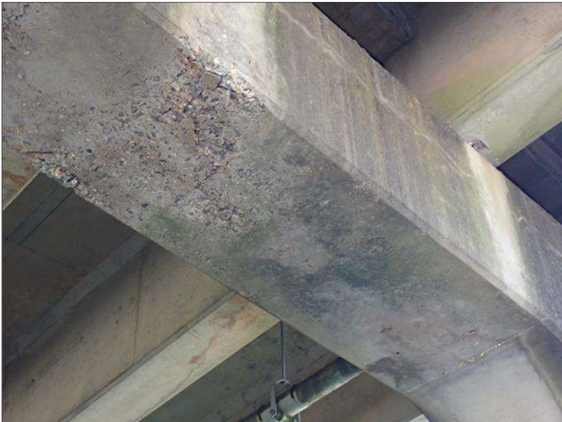
Bent 1 Cap 1: (PAR) underside of cap between columns, delaminations (up to 10 foot x full width) extending into vertical faces (up to 1 foot) with cracks (up to 1/8 inch) with rust stains
