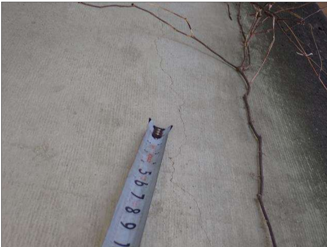
Bent 1 Pile 1: 7 FOOT X UP TO 1/32 INCH VERTICAL CRACK, EAST FACE, BEGINNING AT BOTTOM OF CAP
