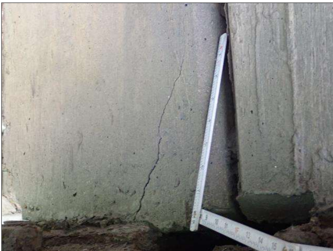
Span 1 Beam 7: at bent 1, both faces, delamination (up to 5 inch x 8 inch) with cracks (up to 1/8 inch)
