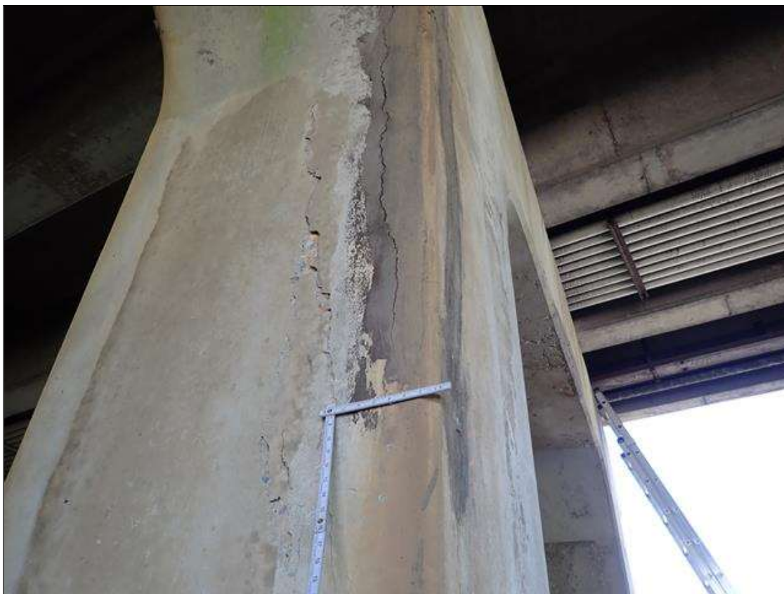
Bent 3 Pile 3: southwest corner, spall/delamination (6 foot x 11 inch x 5 inch x 1 inch deep) with cracks (up to 1/8 inch)
