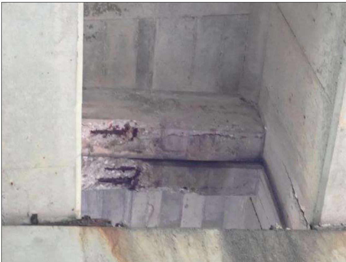
Span 1 Beam 5: (PAR) at bent 1, bay 5 end diaphragm, spall/delamination (full length x full width x up to full height x 1 inch deep) with exposed rusted rebar (approximately 25 percent loss)
