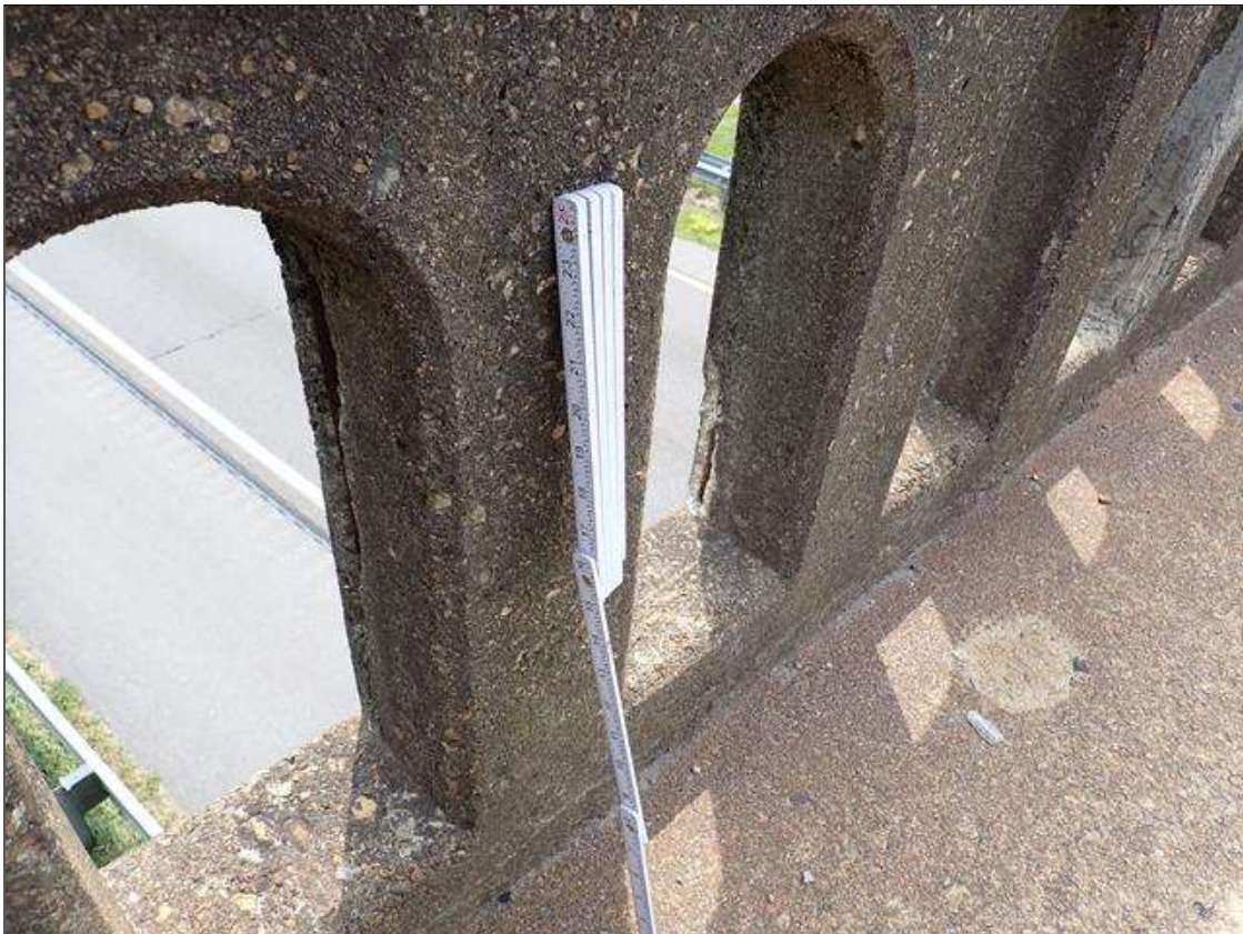
Span 3 Right Bridge Rail: at 6 foot from bent 3, two [2] spalls [up to 18 inch x 2 inch x 3/4 inch deep], both with exposed rusted reinforcing [no loss noted]
