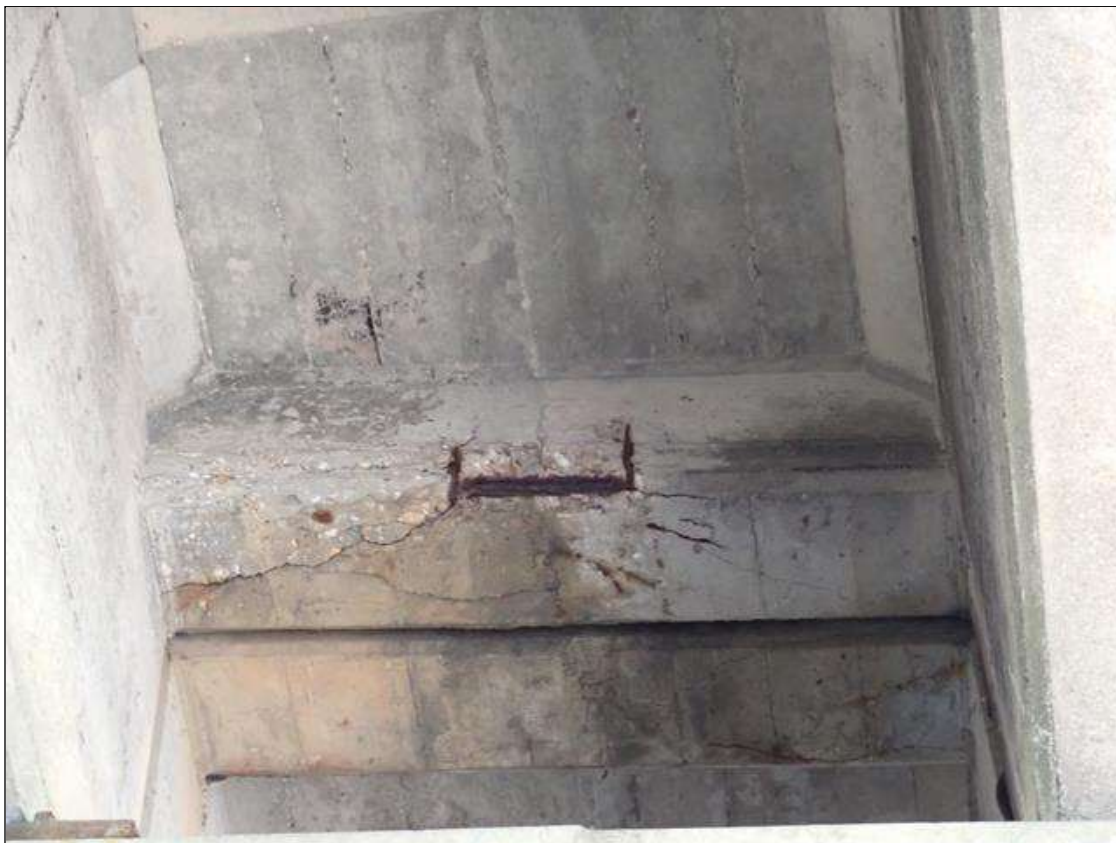
Span 2 Beam 5: (PAR) FULL LENGTH X FULL WIDTH X 10 INCH X 2 INCH DEEP SPALL/DELAMINATION WITH EXPOSED REINFORCING WITH APPROXIMATELY 25 PERCENT LOSS, IN BENT 2 DIAPHRAGM, BAY 5.
