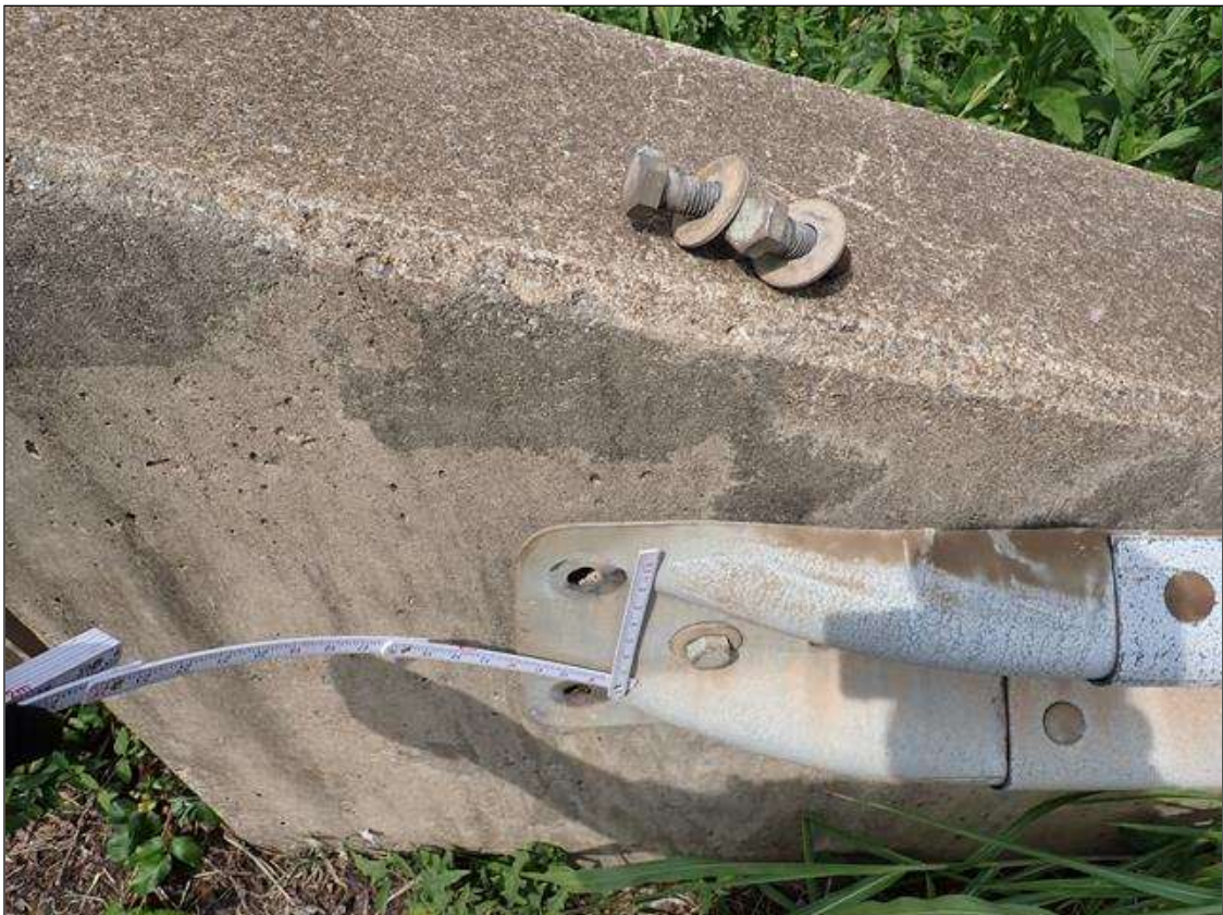
(PAR) northwest guardrail attachment, (2) missing/detached bolts
