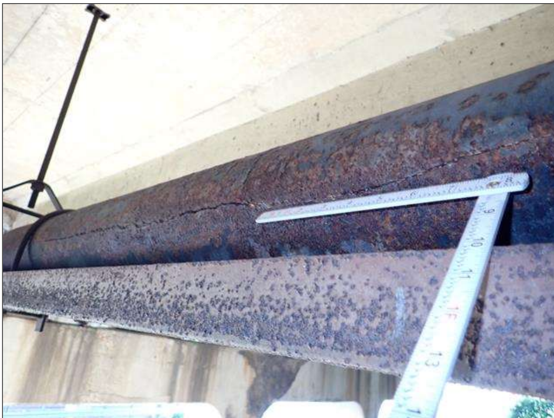
(PAR) span 4, bay 9 utility, near half, broken/cracked
