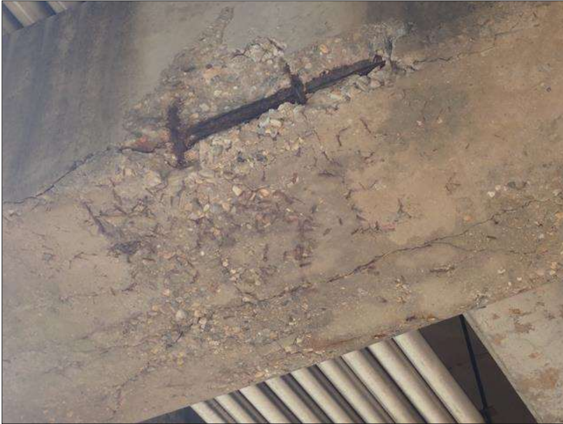
Bent 2 Cap 1: (PAR) [3 FOOT X UP TO 20 INCH X 5 INCH] DEEP SPALL WITH EXPOSED PRIMARY REINFORCING [SECTION LOSS UP TO 1/8 INCH], NORTH AND BOTTOM FACES, BETWEEN PILES 3 AND 4 WITH ADJACENT DELAMINATIONS [UP TO 10 FOOT X FULL WIDTH OF BOTTOM], EXTENDS UP TO FULL HEIGHT OF SOUTH FACE
