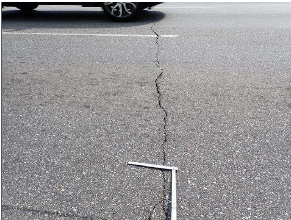
Span 2 Wearing Surface: 58 FOOT X UP TO 1/4 INCH TRANSVERSE CRACK, OVER BENT 1.
