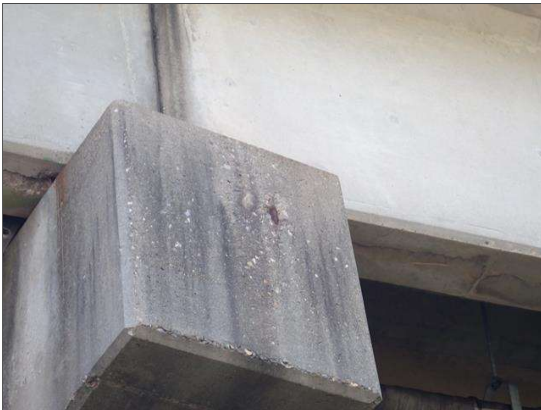
Bent 1 Cap 1: West face, spall [4 inch diameter x 1/2 inch] with exposed rusted reinforcing [no loss noted]
