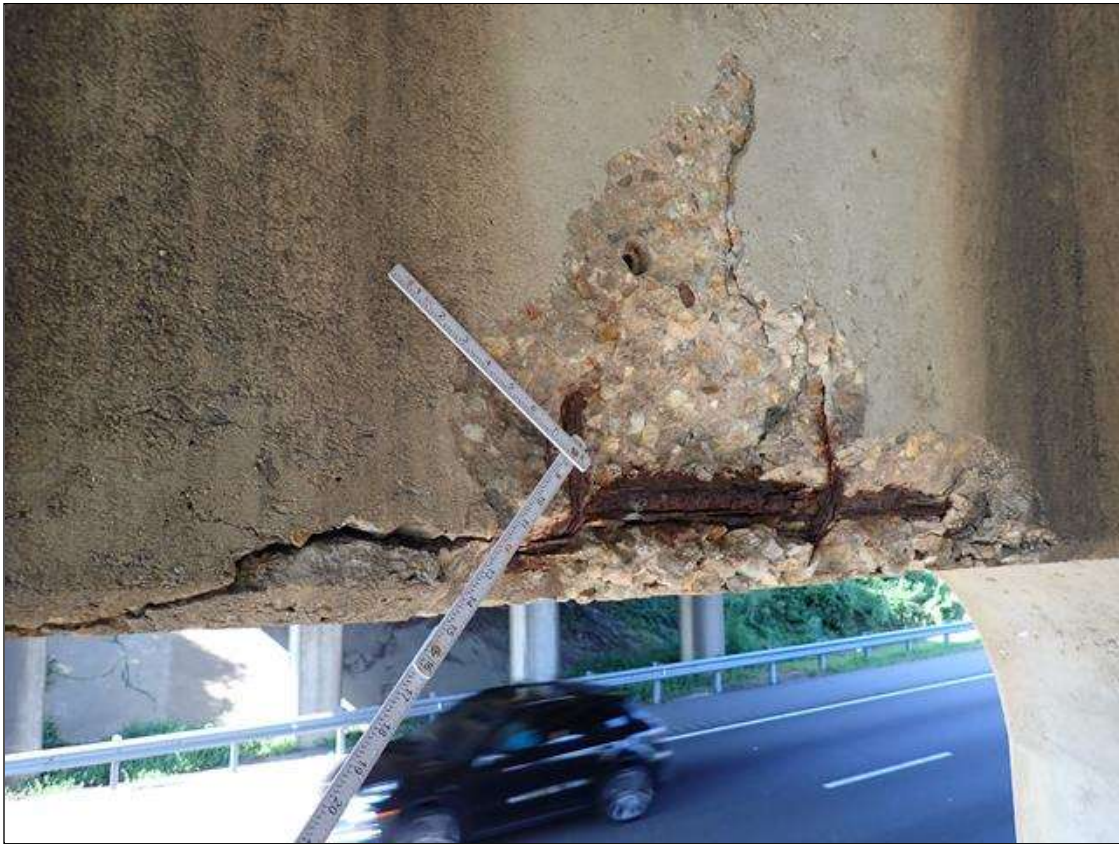
Bent 2 Cap 1: (PAR) [3 FOOT X UP TO 20 INCH X 5 INCH] DEEP SPALL WITH EXPOSED PRIMARY REINFORCING [SECTION LOSS UP TO 1/8 INCH], NORTH AND BOTTOM FACES, BETWEEN PILES 3 AND 4 WITH ADJACENT DELAMINATIONS [UP TO 10 FOOT X FULL WIDTH OF BOTTOM], EXTENDS UP TO FULL HEIGHT OF SOUTH FACE
