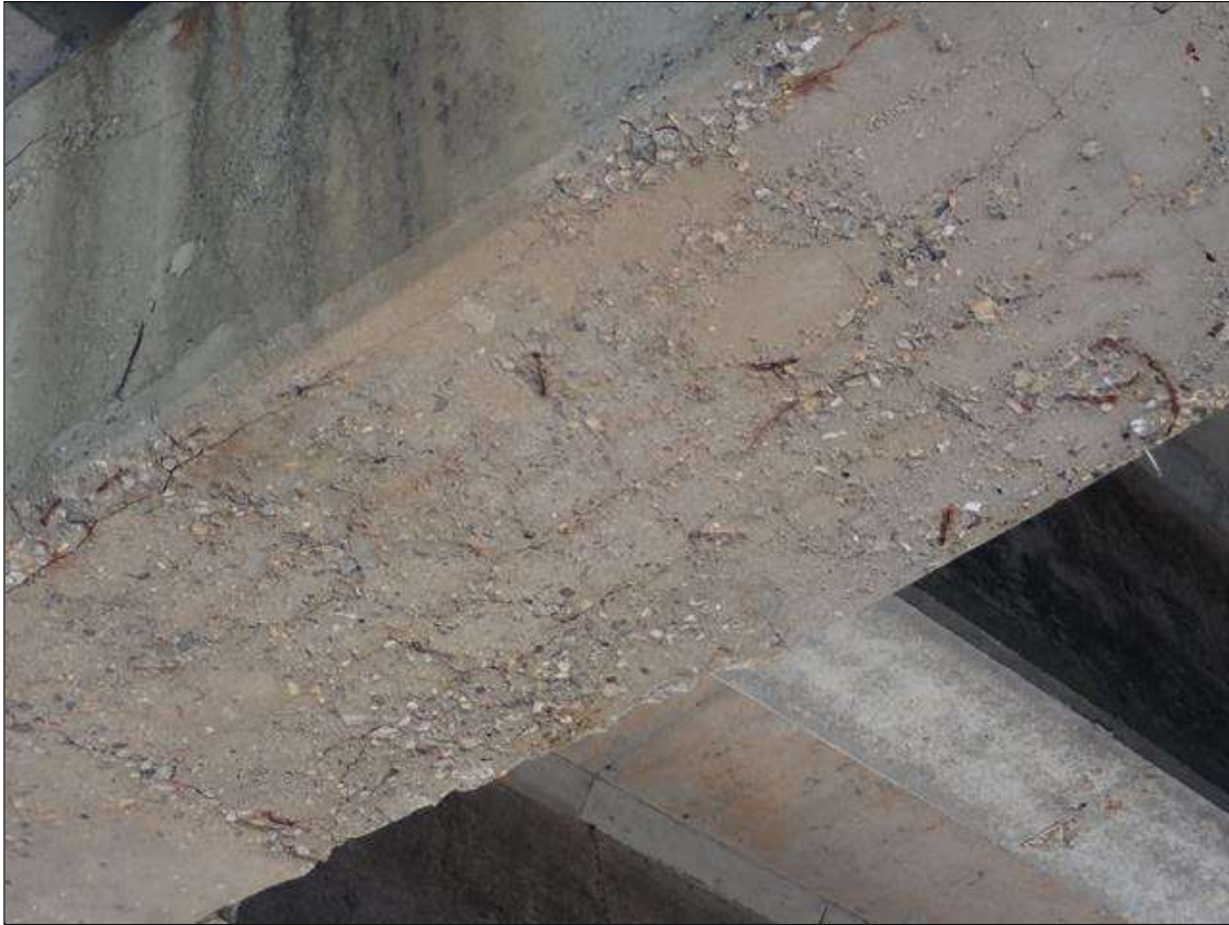
Bent 2 Cap 1: (PAR) 5 FOOT X 1 FOOT X UP TO 3 INCH DEEP SPALL WITH EXPOSED REINFORCING WITH APPROXIMATELY 25 PERCENT LOSS AND MULTIPLE DELAMINATIONS (UP TO 10 FOOT X FULL WIDTH OF BOTTOM X UP TO FULL HEIGHT) WITH CRACKS UP TO 1/8 INCH AND RUST STAINS, SOUTH, NORTH AND BOTTOM FACES, BETWEEN PILES 2 AND 3.
