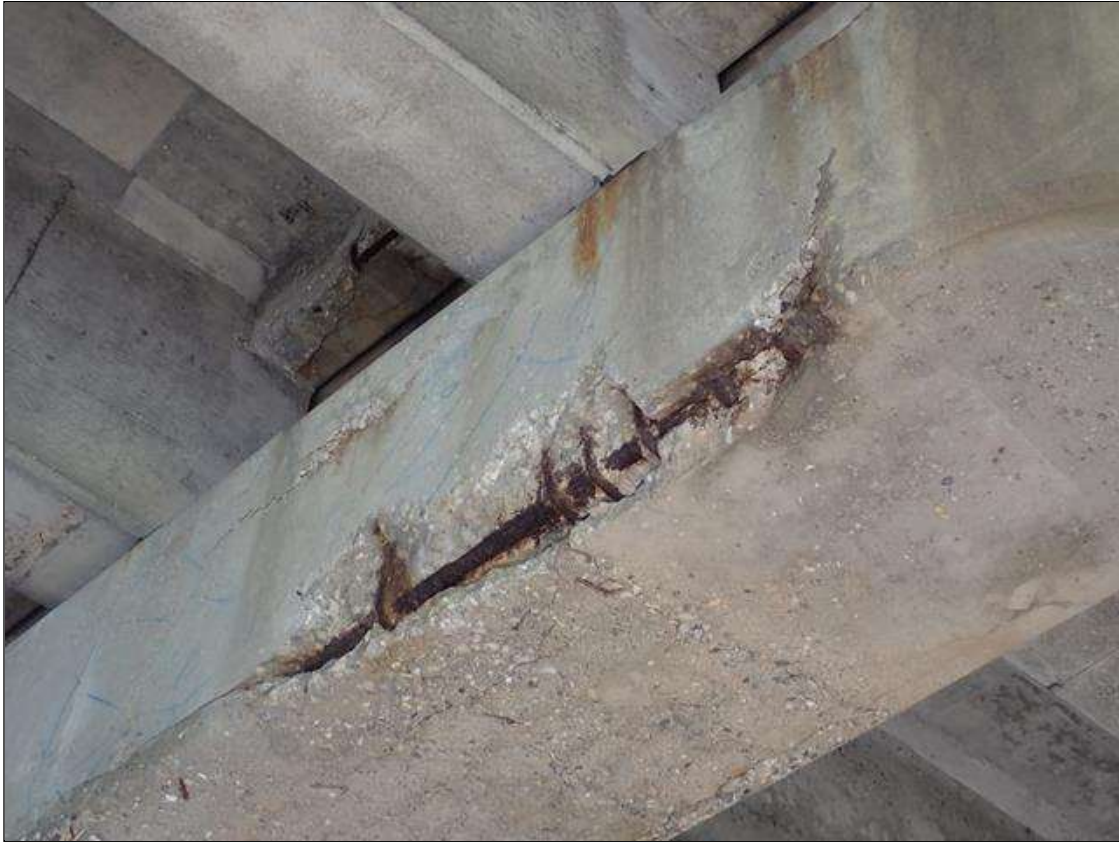
Bent 2 Cap 1: (PAR) 5 FOOT X 1 FOOT X UP TO 3 INCH DEEP SPALL WITH EXPOSED REINFORCING WITH APPROXIMATELY 25 PERCENT LOSS AND MULTIPLE DELAMINATIONS (UP TO 10 FOOT X FULL WIDTH OF BOTTOM X UP TO FULL HEIGHT) WITH CRACKS UP TO 1/8 INCH AND RUST STAINS, SOUTH, NORTH AND BOTTOM FACES, BETWEEN PILES 2 AND 3.
