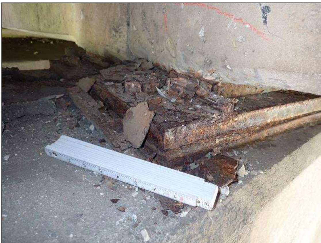
Span 3 Beam 5 - Far Bearing 5: active corrosion with section loss [up to 1/16 inch loss on plates]; anchor bolts, corrosion with section loss [approximately 75 percent remaining]
