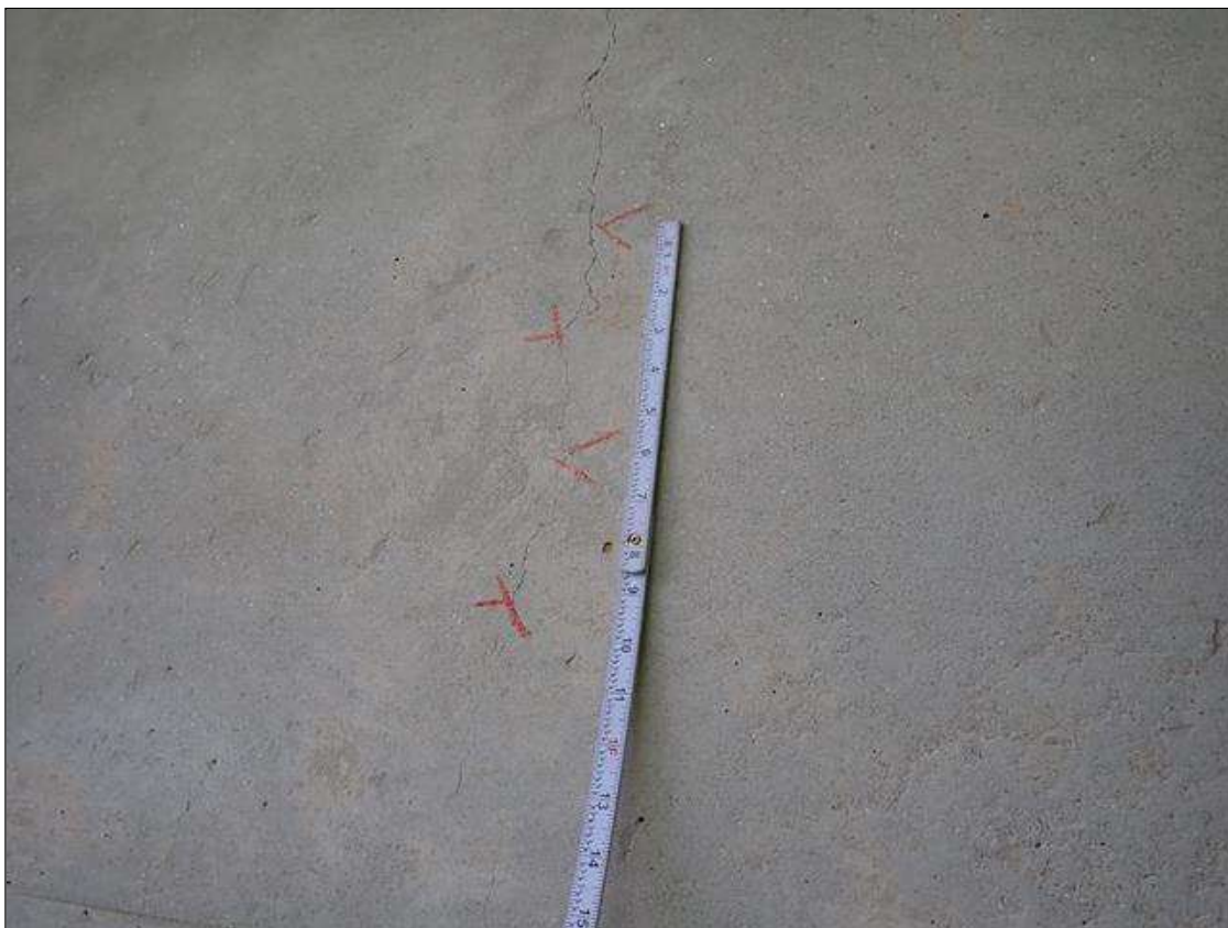
Span 1 Beam 1: along the length of the beam, vertical cracks (up to 1/32 inch x full height) at random
