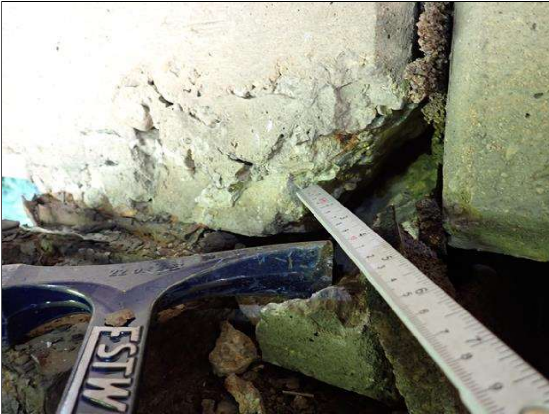
Span 2 Beam 5: at bent 2, east face bottom corner, spall (8 inch x 4 inch x 8 inch x 2 inch deep)
