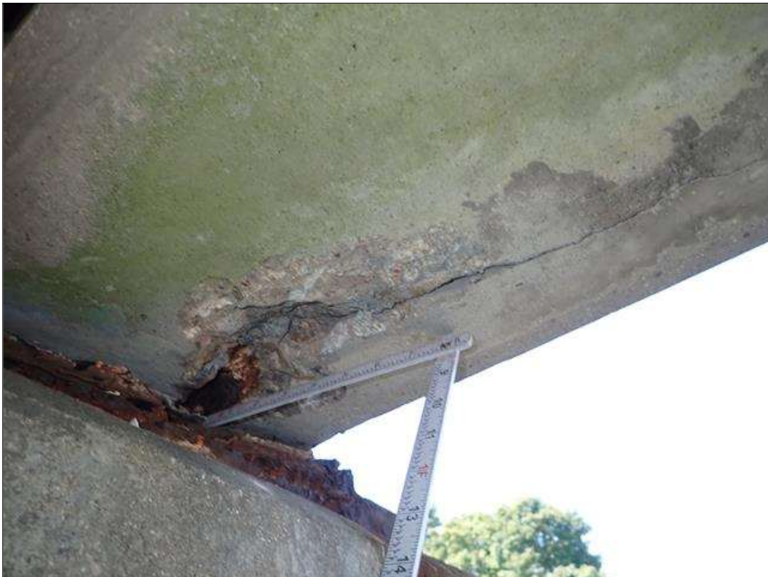
Span 2 Beam 1: at bent 1, underside, spall (9 inch x 4 inch x 1 inch deep) with exposed rusted rebar
