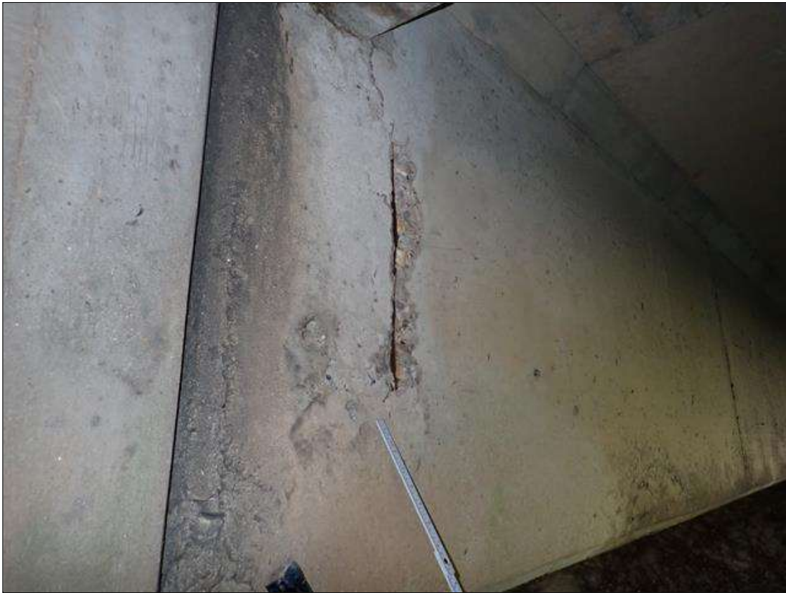
Span 1 Beam 3: (PAR) at bent 1, west face, spall/delamination (8 inch x 24 inch x 1/2 inch deep) with exposed rusted rebar with (approximately 25 percent loss)
