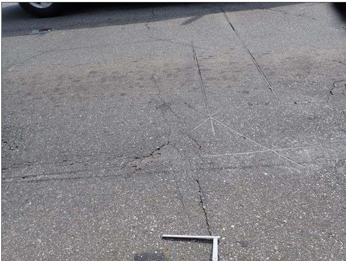
Span 1 Wearing Surface: FULL ROADWAY WIDTH X UP TO 1/8 INCH TRANSVERSE CRACK, OVER END BENT 1.
