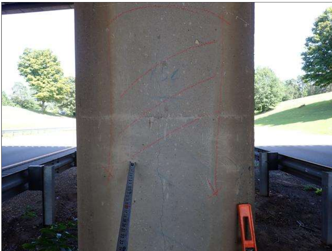
Bent 2 Pile 3: west face at base, delamination/spall (2 foot x 7 foot x 1/2 inch deep) with cracks (up to 1/32 inch)
