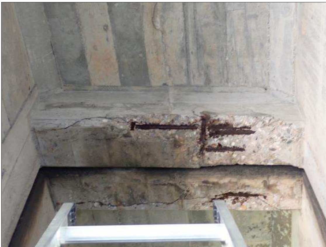
Span 2 Beam 5: (PAR) FULL LENGTH X FULL WIDTH X 8 INCH X 2 INCH DEEP SPALL WITH EXPOSED REINFORCING WITH APPROXIMATELY 25 PERCENT LOSS, IN BENT 1 DIAPHRAGM, BAY 5.
