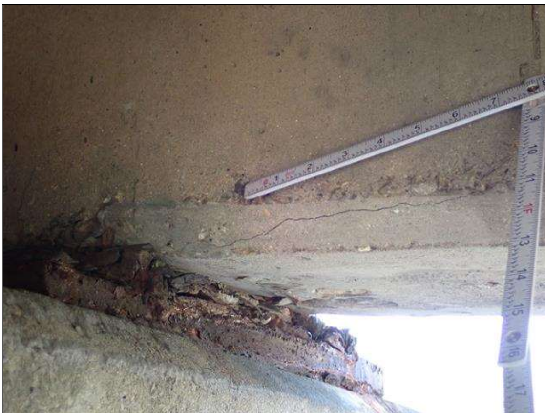
Span 3 Beam 1: at bent 2, east face at bottom, longitudinal crack (1/32 inch x 1 foot)
