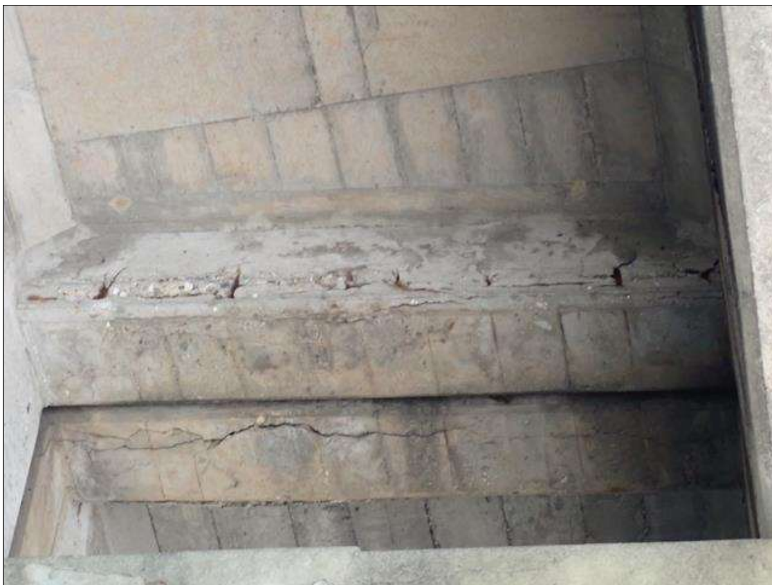
Span 2 Beam 6: FULL LENGTH X FULL WIDTH X 12 INCH X 2 INCH DEEP SPALL/DELAMINATION IN BAY 6 DIAPHRAGM AT BENT 2.
