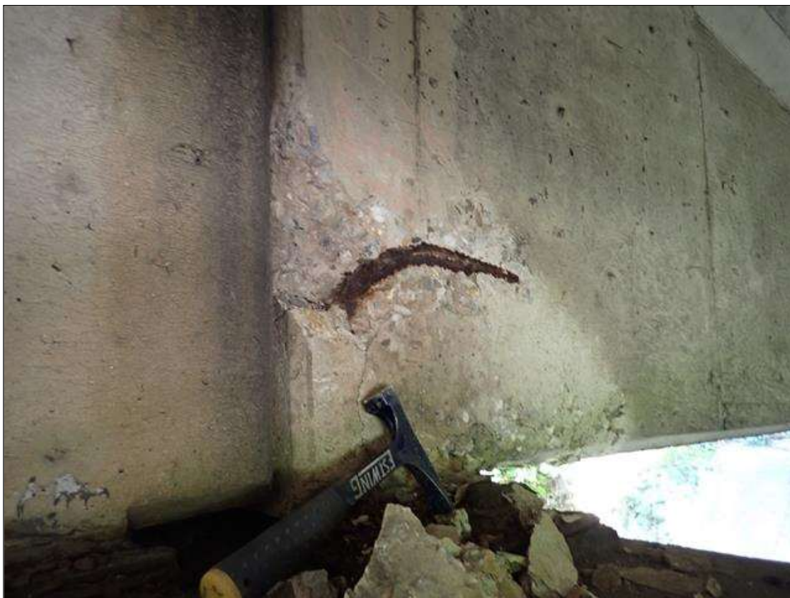
Span 4 Beam 2: (PAR) at near end, east face, spall/delamination [18 inch x 18 inch x up to 2 inch deep] with exposed rusted reinforcing [section loss up to 1/16 inch]
