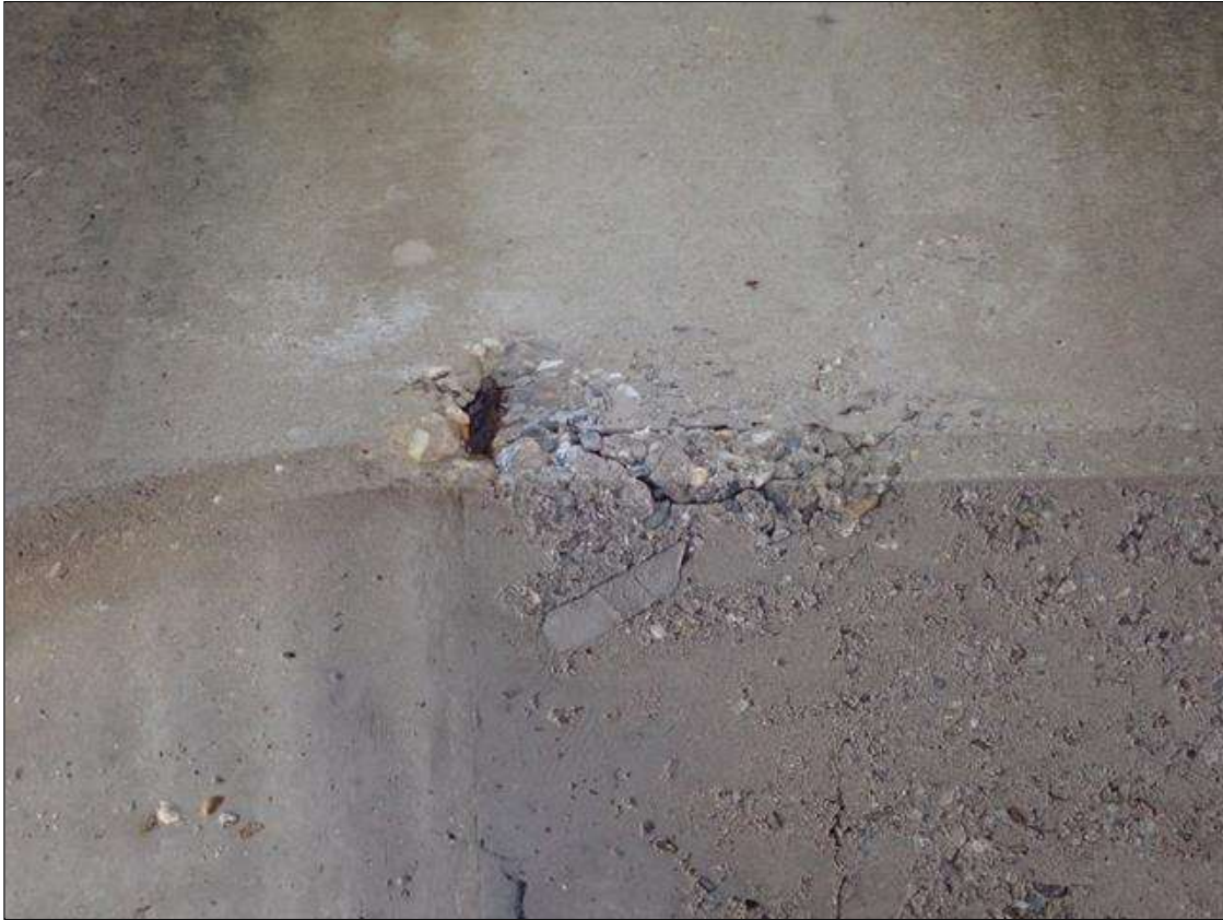
Bent 2 Cap 1: (PAR) 6 INCH DIAMETER X 1 INCH DEEP SPALL WITH EXPOSED REINFORCING WITH APPROXIMATELY 25 PERCENT LOSS, SOUTH FACE, UNDER BEAM 2.
