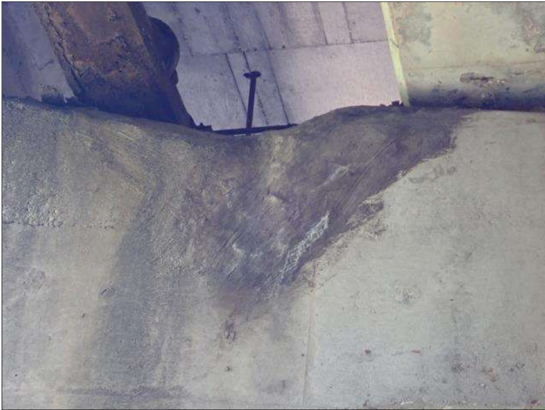
Bent 3 Cap 1: BENT 3 CAP NORTH FACE BAY 9. HAS A PATCHED AREA 3 FOOT X 2 FOOT WITH SCATTERED HAIRLINE CRACKS WITH EFFLORESCENCE VISIBLE
