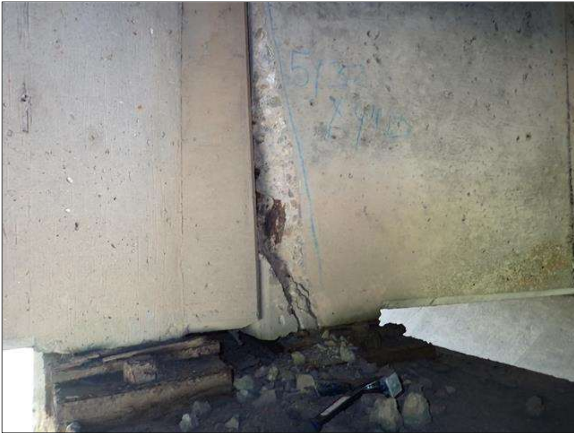
Span 4 Beam 6: (PAR) SPAN 4 BEAM 6 EAST WEB OVER BENT 3. HAS A CRACK/SPALL AND DELAMINATED AREA WITH REBAR WITH APPROXIMATELY 25 PERCENT LOSS AND RUST STAINS VISIBLE. AREA IS: 5 INCH X 32 INCH X 4 INCH DEEP.
