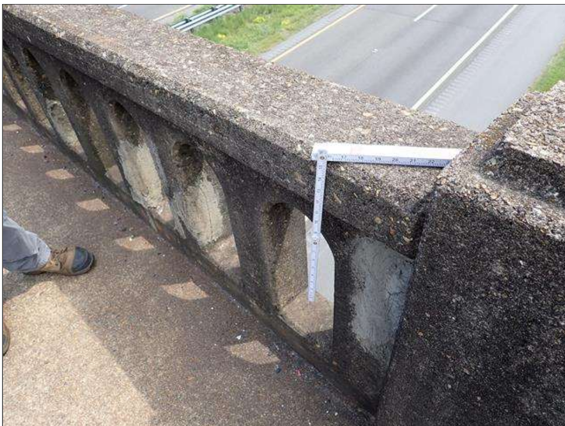
Span 2 Right Bridge Rail: SPAN 2 RIGHT RAIL HAS (11) PATCHED AREAS UP TO 8 INCH X 1 FOOT WITH HAIRLINE CRACKS.
