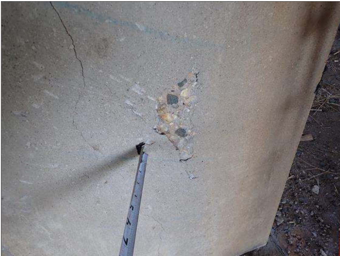
Bent 2 Pile 3: west face at base, delamination/spall (2 foot x 7 foot x 1/2 inch deep) with cracks (up to 1/32 inch)
