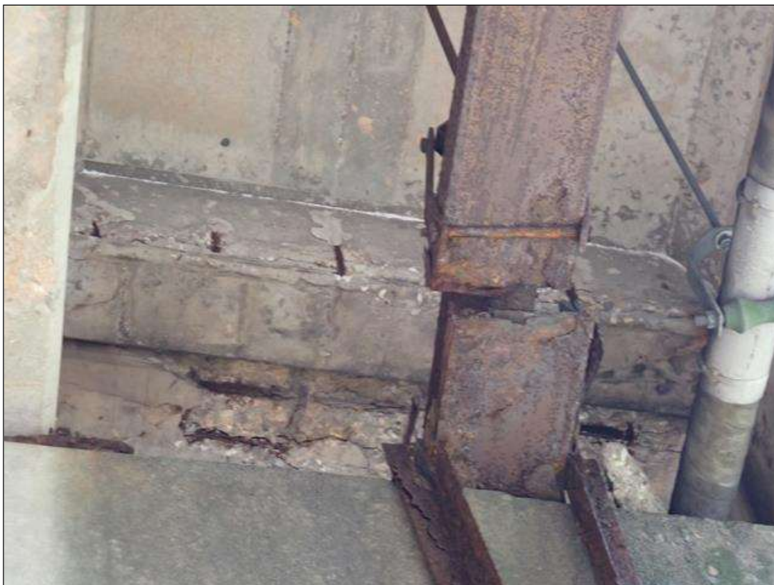
Span 2 Beam 9: FULL LENGTH X FULL WIDTH X 12 INCH X 1 INCH DEEP SPALL/DELAMINATION WITH EXPOSED REINFORCING, IN BENT 2 DIAPHRAGM, BAY 9.
