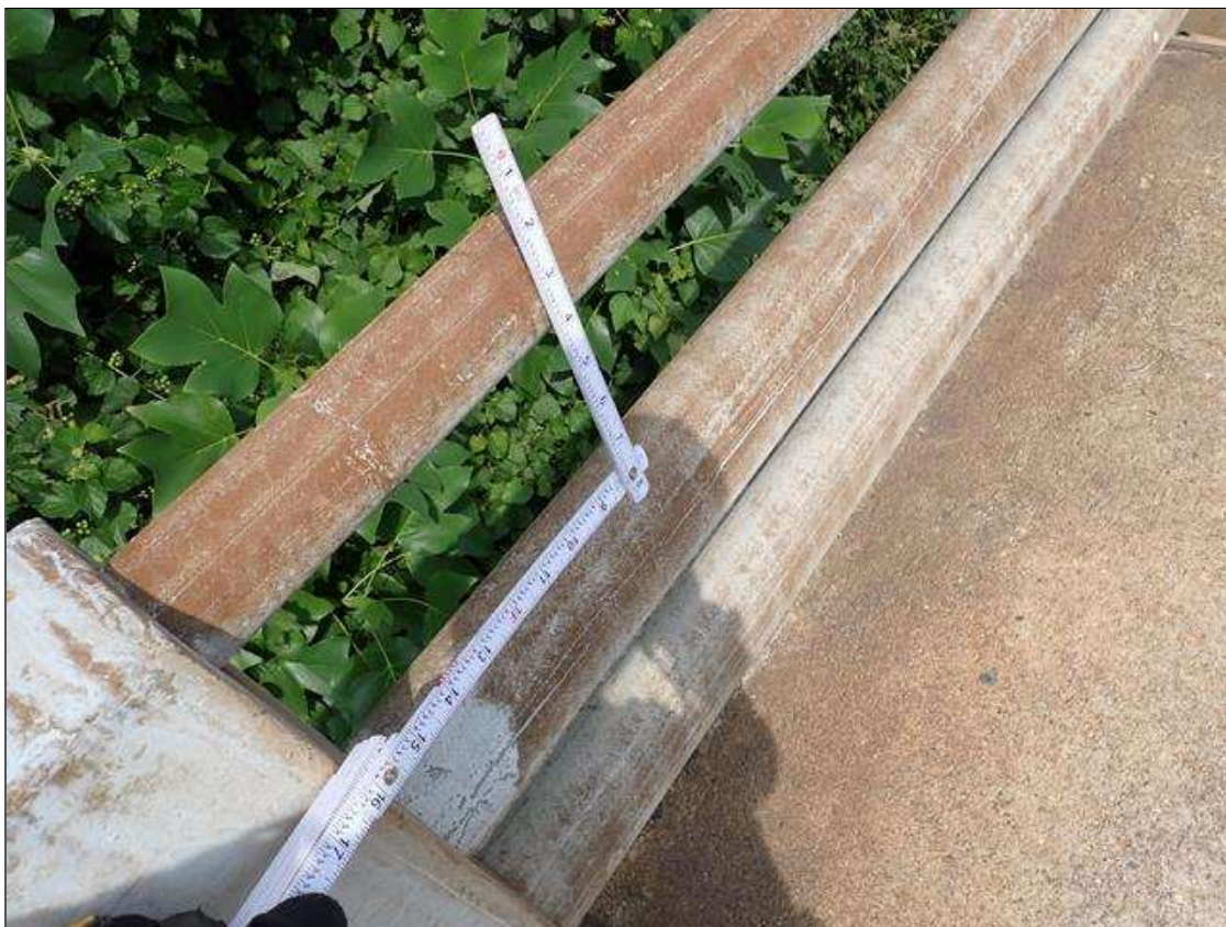
Span 1 Left Bridge Rail: surface rust at random
