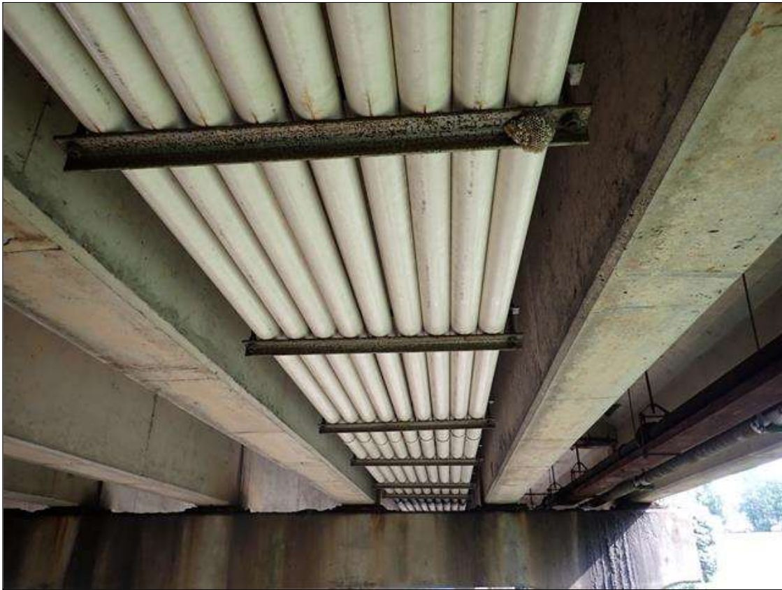
bay 8, (9) pvc pipes (4 inch diameter)
