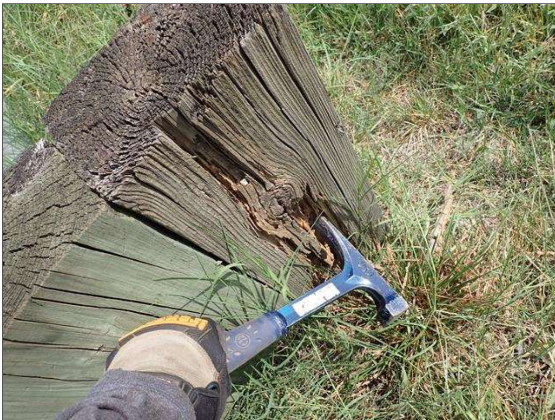
(PAR) southeast guardrail, timber posts 7, 12 and 14, decay/section loss (up to full width x full height x full depth)
