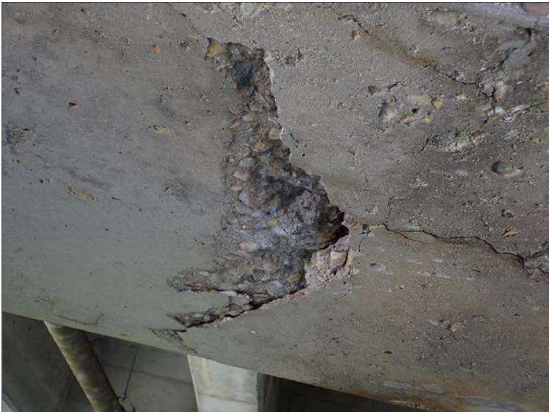
Bent 3 Cap 1: (PAR) underside of cap between all piles, delaminations/spalls [up to 8 foot x full width x 2 inch deep], extend up vertical face (4 inch) with cracks (up to 1/4 inch)
