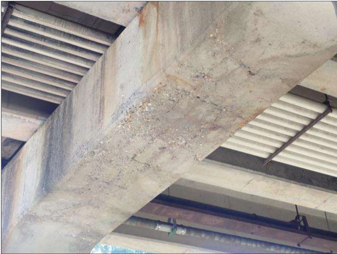
Bent 1 Cap 1: (PAR) underside of cap between columns, delaminations (up to 10 foot x full width) extending into vertical faces (up to 1 foot) with cracks (up to 1/8 inch) with rust stains
