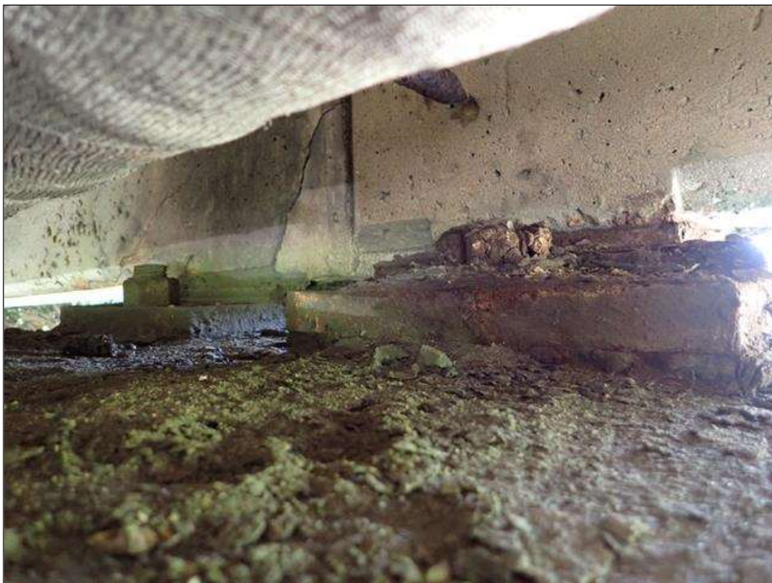
interior bearing assembly
