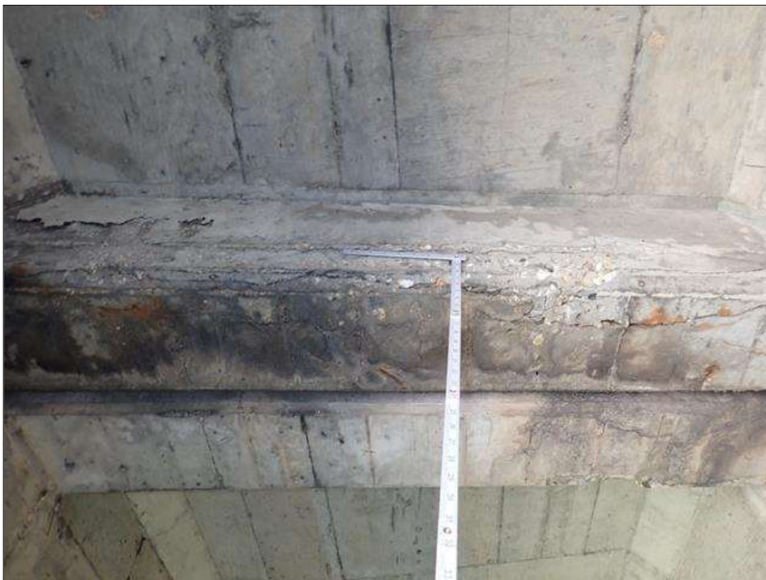
Span 3 Beam 2: (PAR) at bent 3, bay 2 end diaphragm, delamination (full width x 8 inch) with cracks (up to 1/2 inch deep) with rust stains
