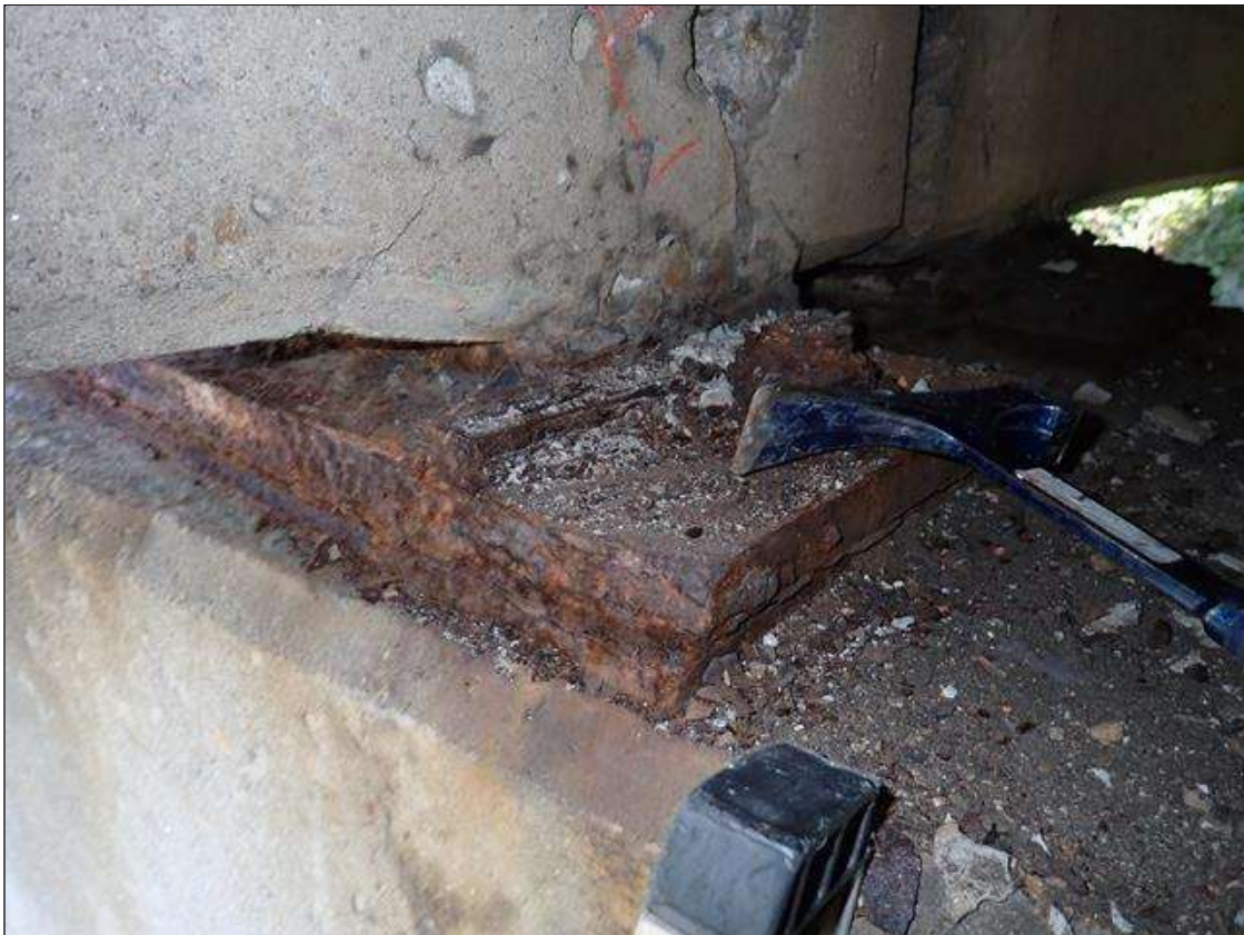
Span 3 Beam 1 - Far Bearing 1: active corrosion with section loss [up to 1/8 inch loss on plates]; anchor bolts, corrosion with section loss [approximately 75 percent remaining]
