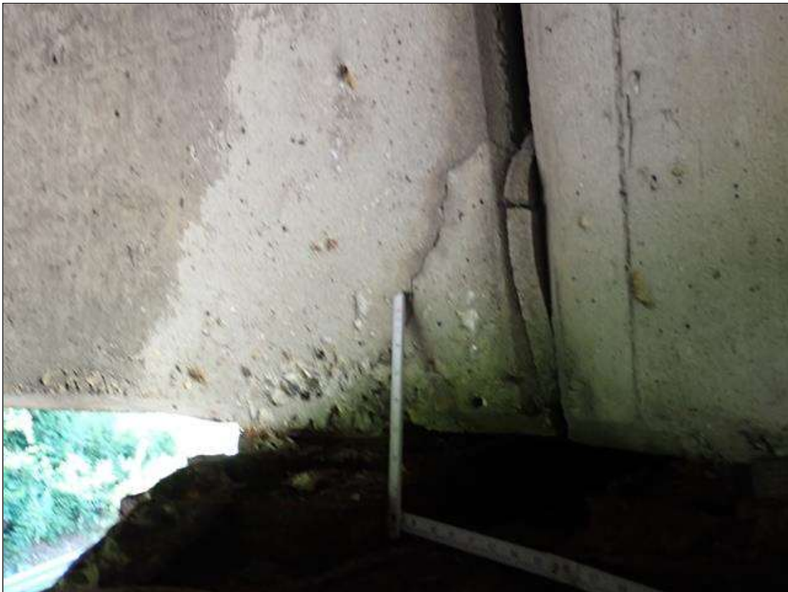
Span 2 Beam 3: at bent 2, east face, delamination (7 inch x 8 inch) with cracks (up to 1/16 inch)
