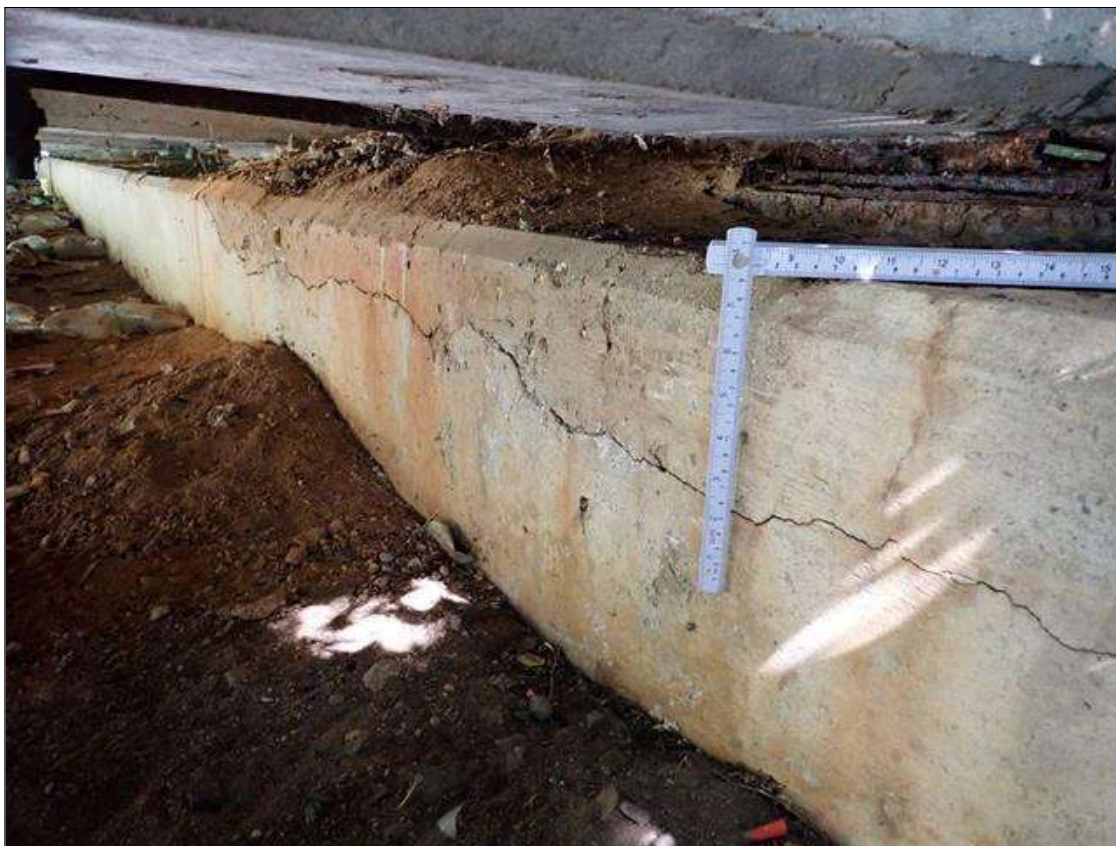
End Bent 2 Cap 1: below bay 9, delamination (8 foot x 5 inch x 5 inch) with cracks (up to 3/16 inch)
