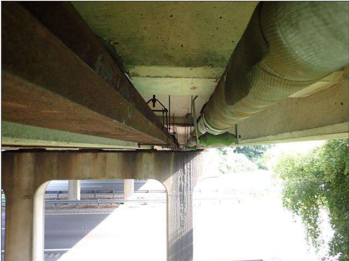
bay 9, cast iron pipe utility (6 inch diameter) and gas line (4 inch diameter)
