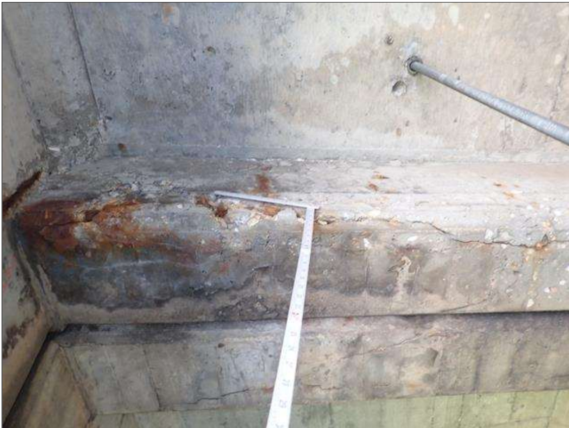
Span 3 Beam 1: (PAR) at bent 3, bay 1 end diaphragm, delamination (full width x full height) with cracks (up to 1/2 inch deep) with rust stains
