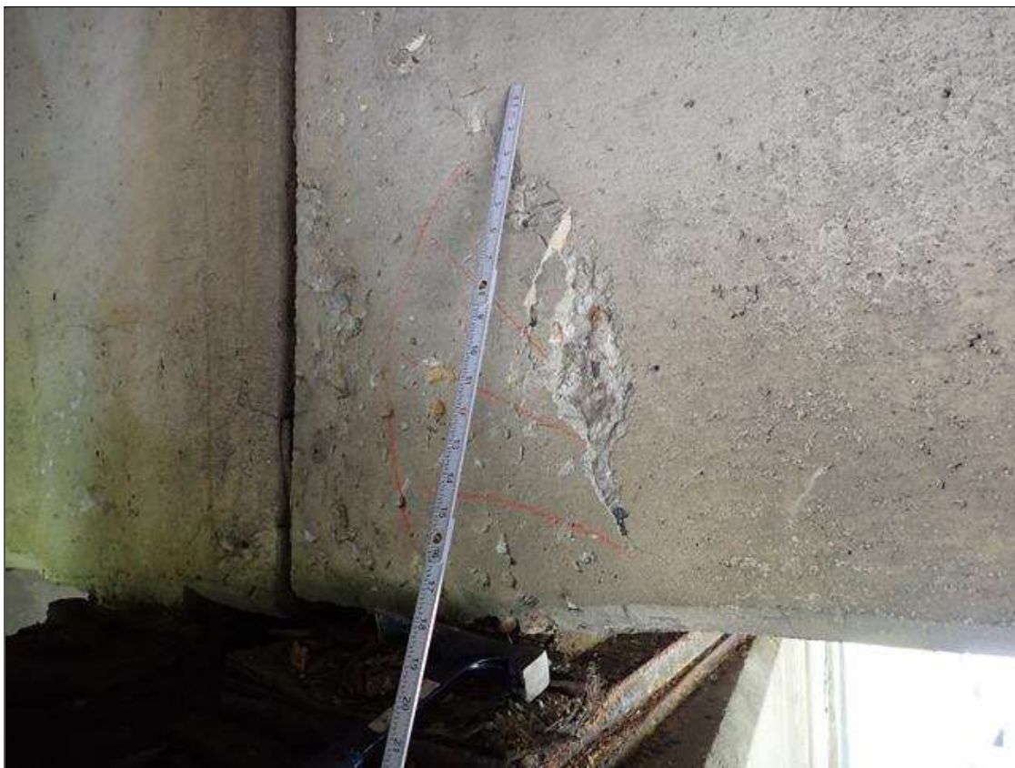
Span 3 Beam 5: at bent 3, west face, spall/delamination (1 foot x 1.5 foot x 1 inch deep)
