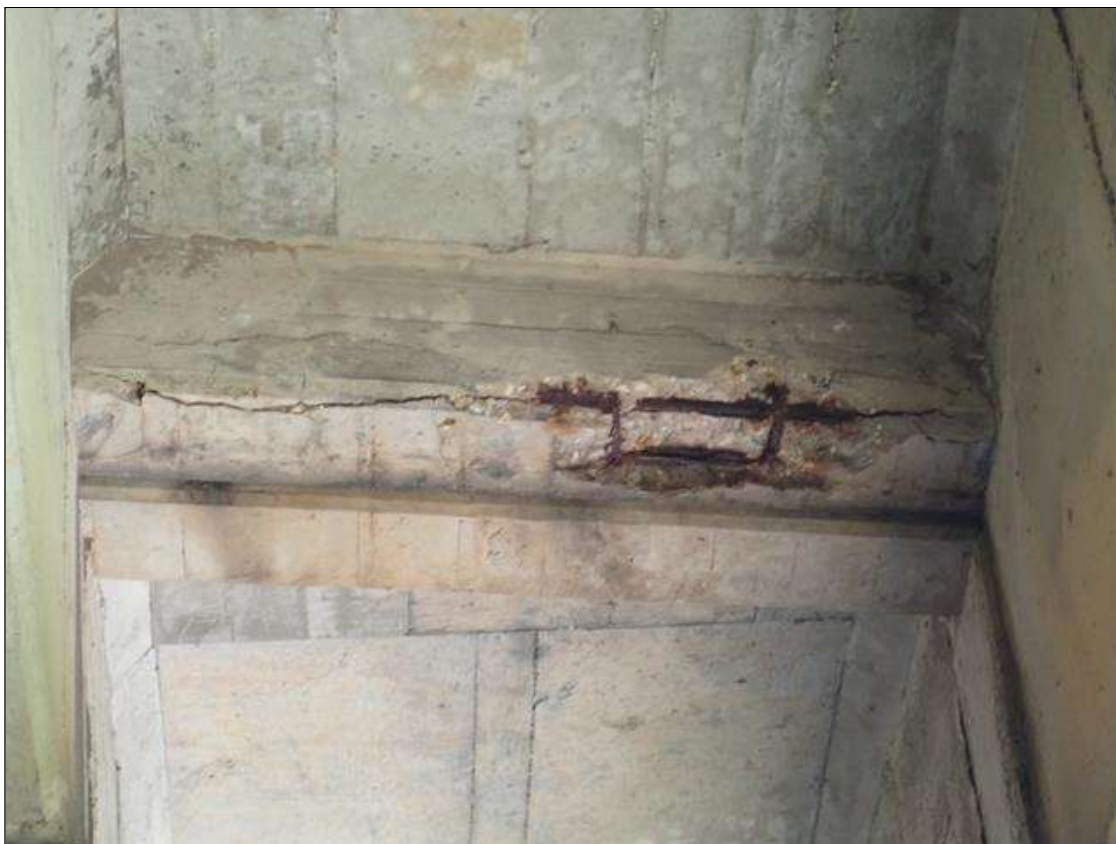
Span 1 Beam 7: (PAR) at bent 1, bay 7 end diaphragm, spall/delamination (full length x full width x up to full height x 1 inch deep) with exposed rusted rebar (approximately 25 percent loss)
