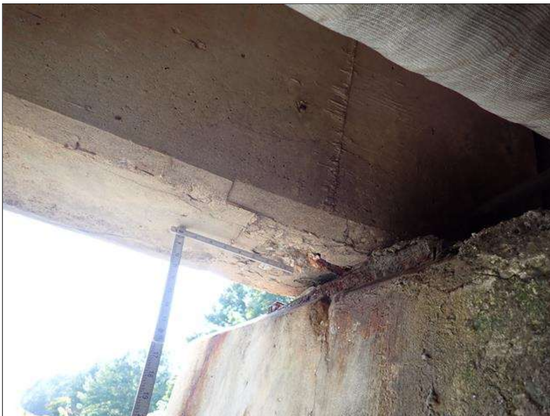
Span 2 Beam 10: underside at bent 1, spall/delamination [1.5 foot x full width x 1 inch deep] with exposed rusted rebar
