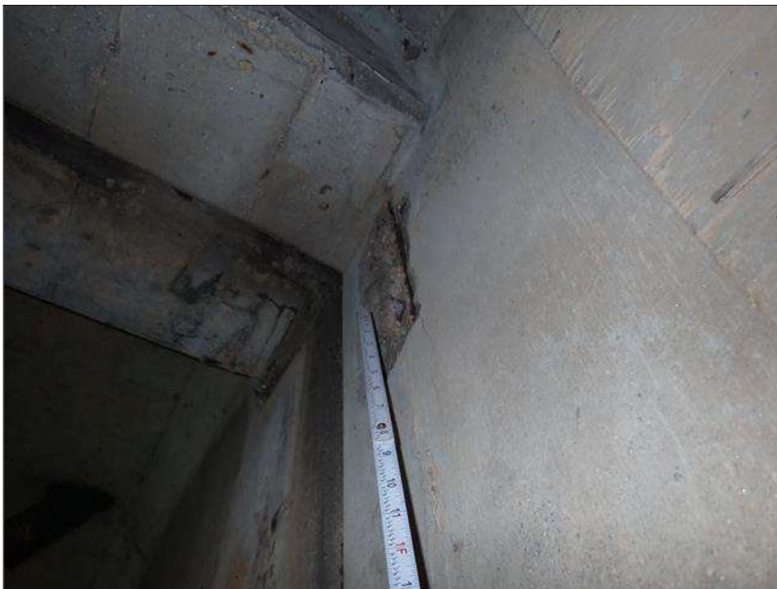
Span 2 Beam 1: at bent 1, east face, spall/delamination (6 inch x 11 inch x 1/2 inch deep) with exposed rusted rebar
