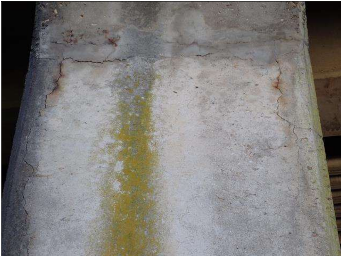
Bent 1 Pile 4: (PAR) (2)- UP TO 5 FOOT X 1/32 INCH VERTICAL CRACKS WITH RUST STAIN, EAST FACE, BEGINNING AT BOTTOM OF CAP.
