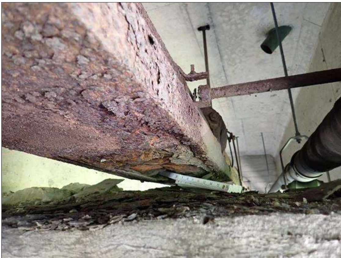
(PAR) at bent 3, utility platform, corrosion with section loss (up to 100 percent loss) with corrosion holes (up to 3 inch diameter); hanger connection, corrosion with section loss (up to 100 percent loss)
