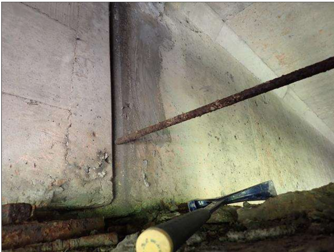
Span 4 Beam 9: East face at near end, patched area [16 inch x 8 inch]
