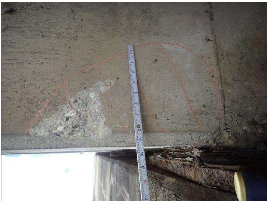
Span 2 Beam 6: at bent 1, west face, delamination/spall (18 inch x 9 inch x 1/2 inch deep)
