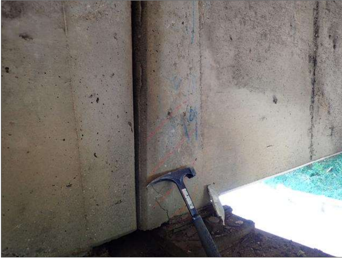
Span 2 Beam 8: West face at far end, delamination [10 inch x full height]
