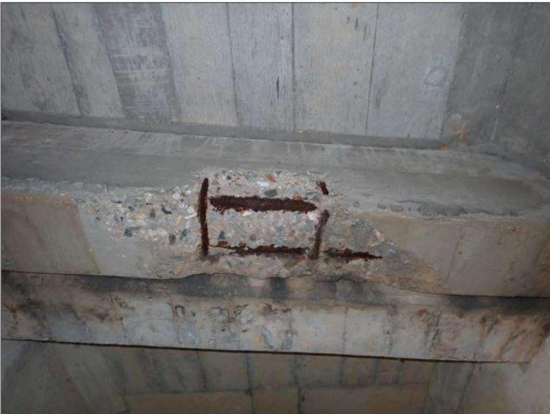
Span 2 Beam 3: (PAR) FULL LENGTH X FULL WIDTH X 8 INCH X 2 INCH DEEP SPALL/DELAMINATION WITH EXPOSED RUSTED REBAR WITH APPROXIMATELY 25 PERCENT LOSS IN BAY 3 DIAPHRAGM AT BENT 1.
