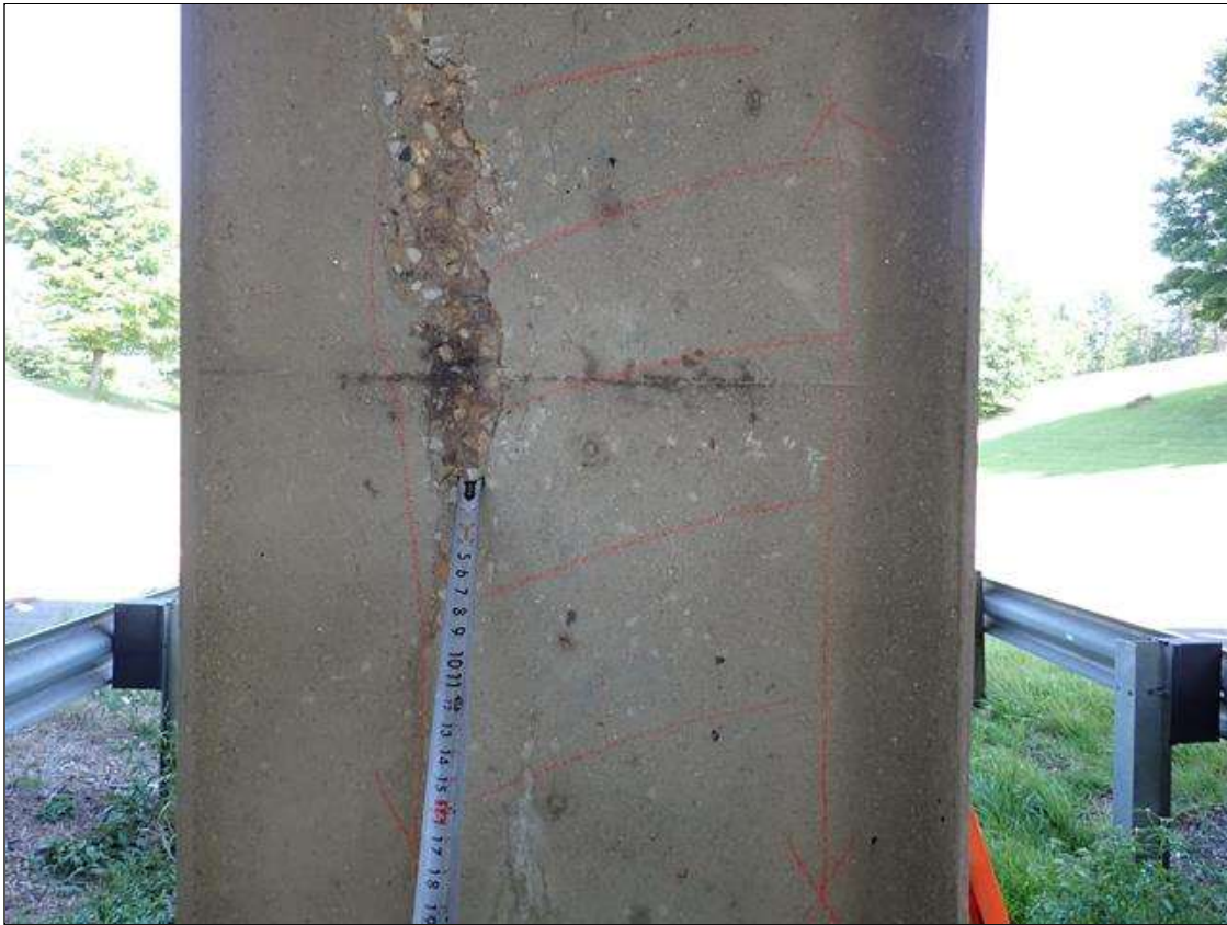
Bent 2 Pile 4: west face, spall/delamination (2 foot x full height x 1/2 inch deep) with cracks (up to 1/32 inch) some with efflorescence
