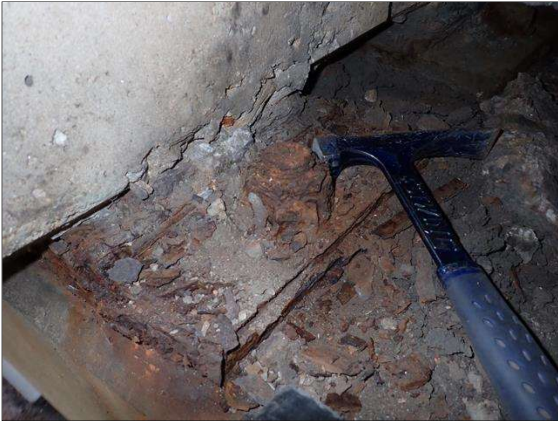
Span 3 Beam 2 - Near Bearing 2: active corrosion with section loss [up to 1/8 inch loss on plates]; anchor bolts, corrosion with section loss [approximately 75 percent remaining]
