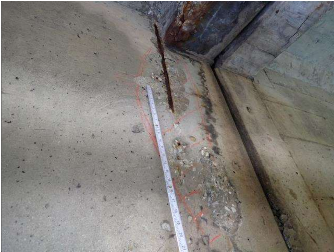
Span 3 Beam 1: (PAR) 10 INCH X 39 INCH X 1 INCH DEEP SPALL/DELAMINATION WITH EXPOSED REINFORCING WITH APPROXIMATELY 25 PERCENT LOSS, EAST FACE OF WEB, AT BENT 3.
