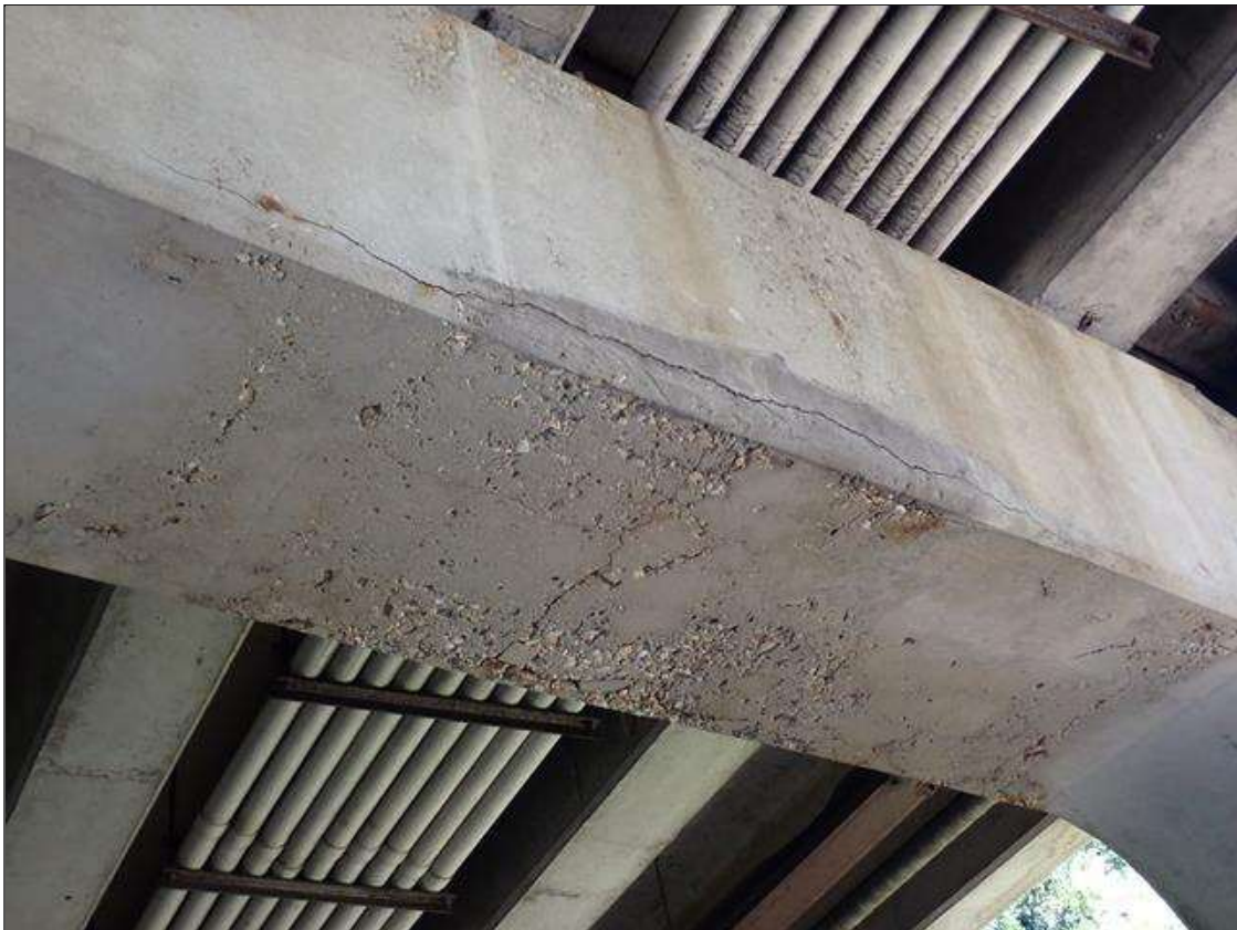
Bent 3 Cap 1: (PAR) underside of cap between all piles, delaminations/spalls [up to 8 foot x full width x 2 inch deep], extend up vertical face (4 inch) with cracks (up to 1/4 inch)
