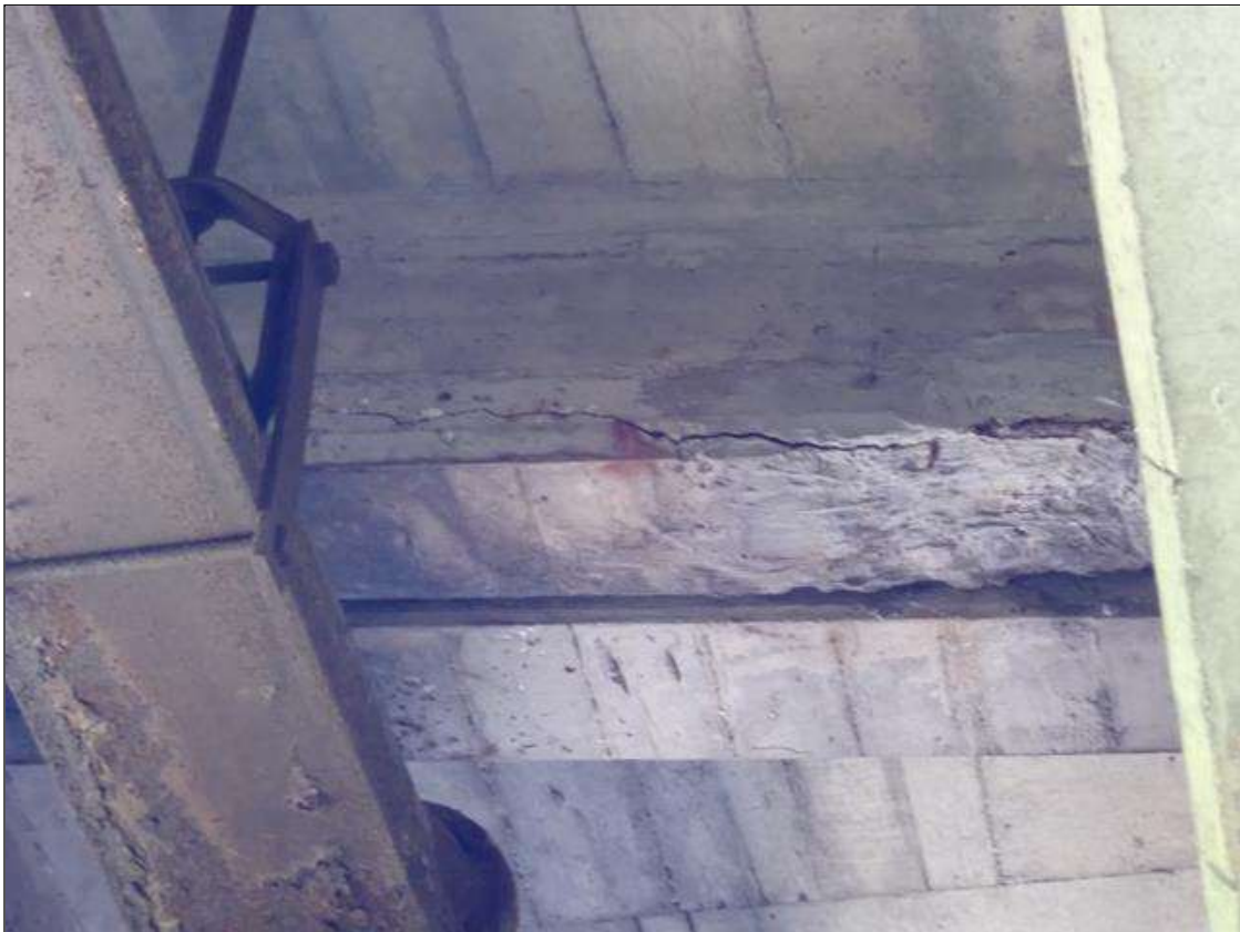
Span 4 Beam 9: (PAR) FULL LENGTH X 8 INCH X FULL WIDTH FAILED PATCH/DELAMINATION WITH CRACKS (UP TO 1/4 INCH) WITH RUST STAINS, IN BENT 3 DIAPHRAGM, BAY 9
