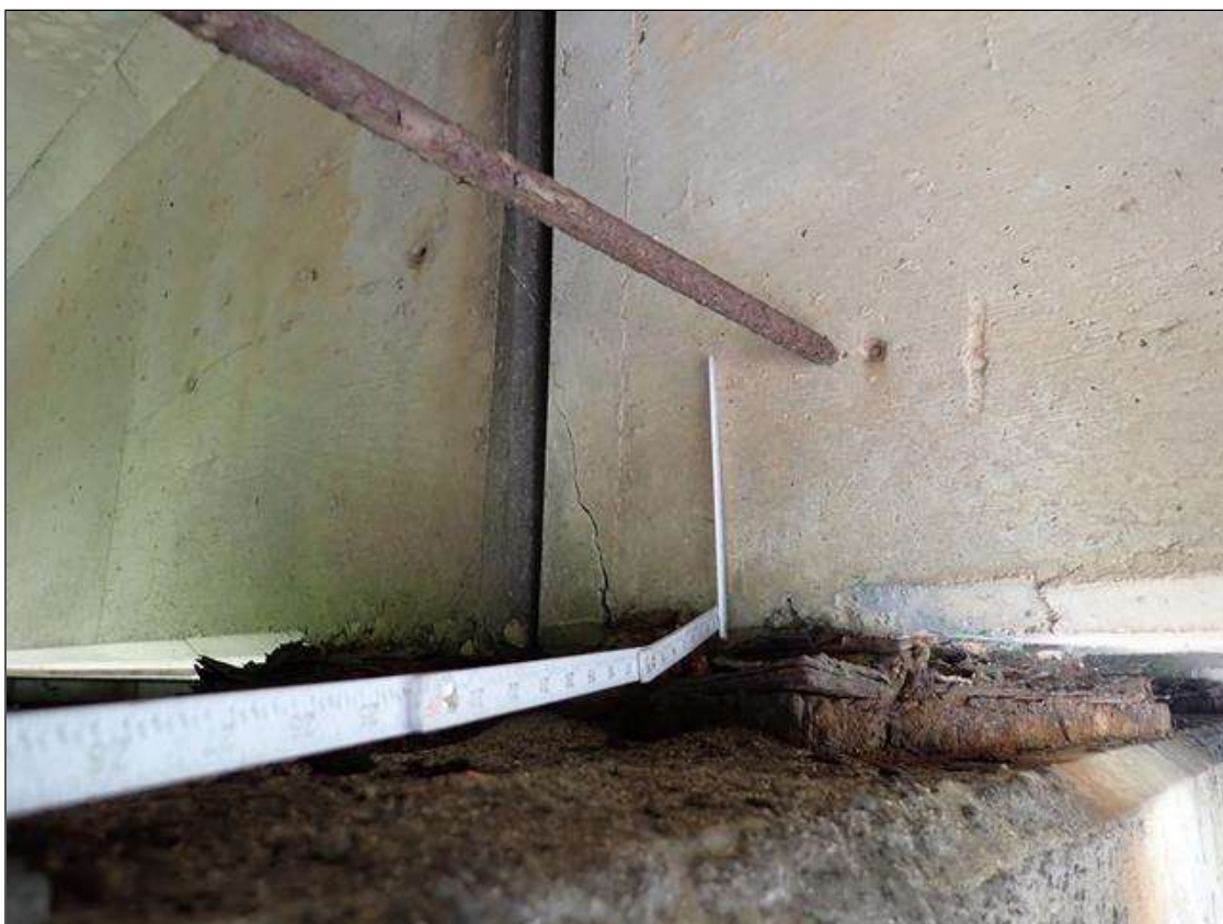
Span 2 Beam 9: at bent 1, delamination (9 inch x 3 inch) with cracks (up to 1/8 inch)
