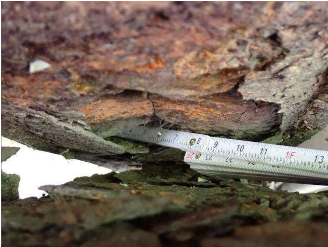
(PAR) at bent 3, utility platform, corrosion with section loss (up to 100 percent loss) with corrosion holes (up to 3 inch diameter); hanger connection, corrosion with section loss (up to 100 percent loss)
