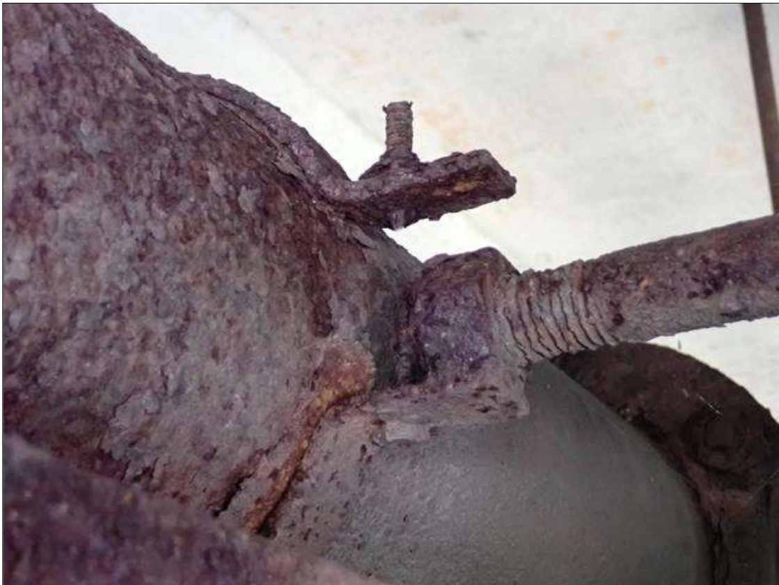
(PAR) at bent 3, utility platform, corrosion with section loss (up to 100 percent loss) with corrosion holes (up to 3 inch diameter); hanger connection, corrosion with section loss (up to 100 percent loss)
