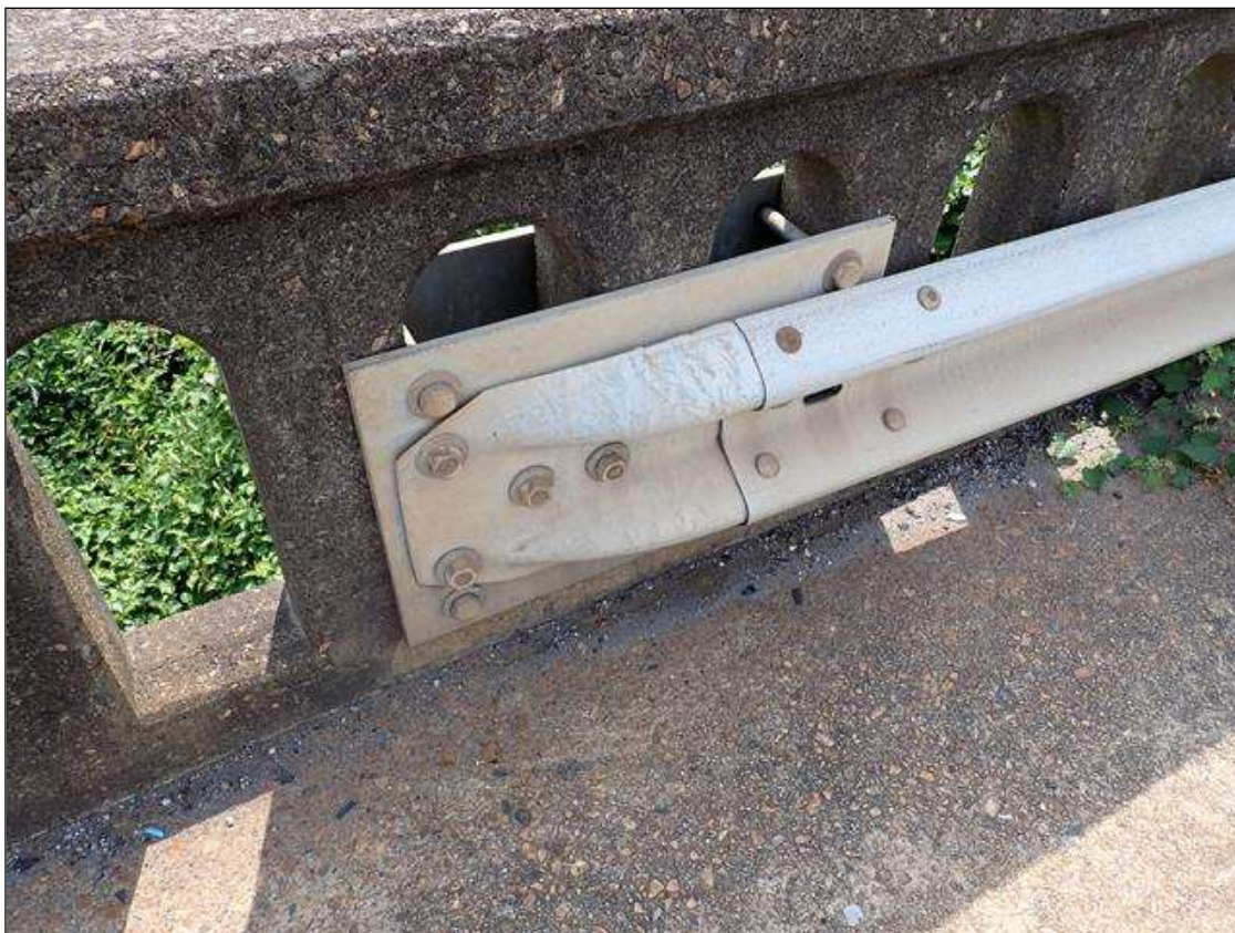
southeast guardrail attachment
