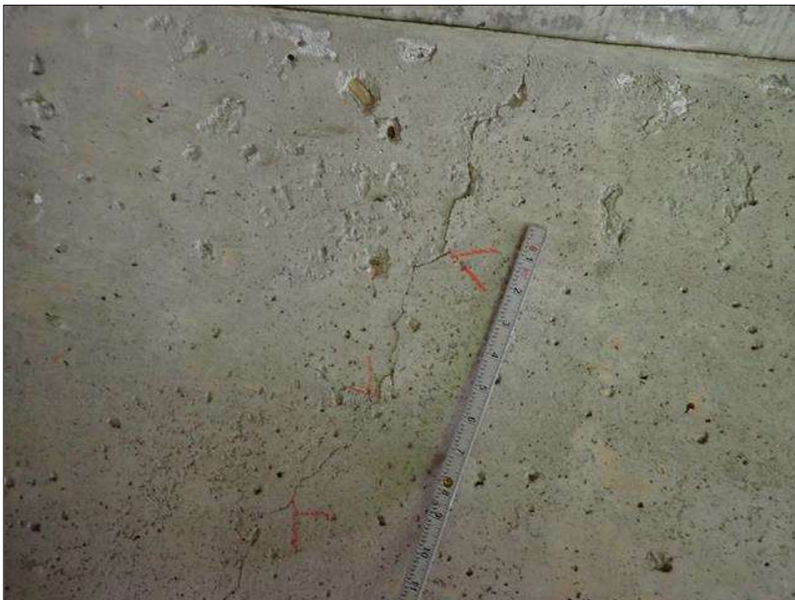
Span 1 Beam 9: along the length of the beam, vertical cracks (up to 1/32 inch x full height) at random
