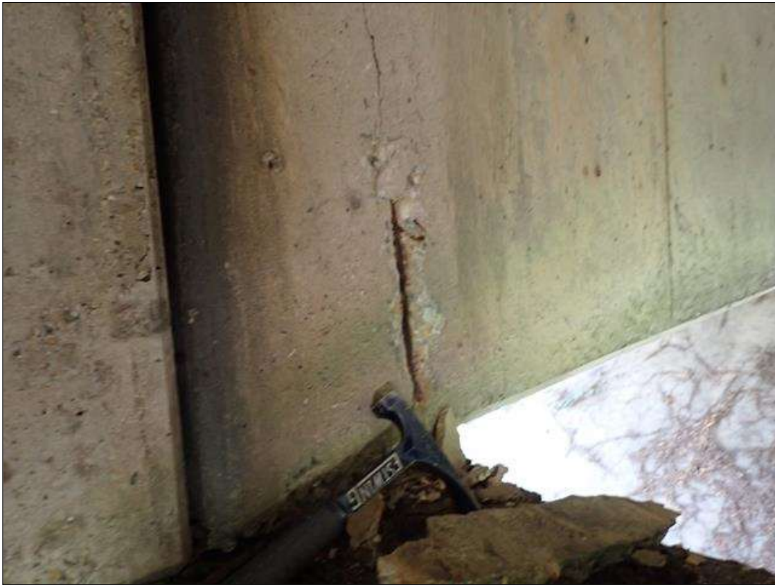
Span 1 Beam 6: (PAR) at bent 1, west face, spall/delamination (5 inch x 30 inch x 1/2 inch deep) with exposed rusted rebar (approximately 25 percent loss)
