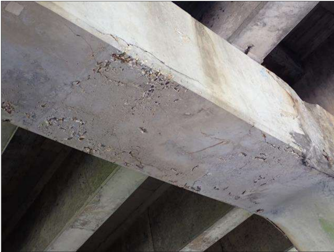
Bent 3 Cap 1: (PAR) underside of cap between all piles, delaminations/spalls [up to 8 foot x full width x 2 inch deep], extend up vertical face (4 inch) with cracks (up to 1/4 inch)
