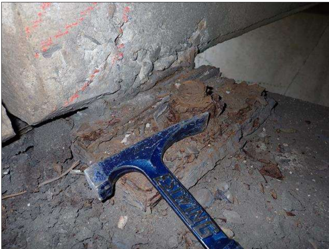
Span 4 Beam 3 - Near Bearing 3: active corrosion with section loss [up to 1/8 inch loss on plates]; anchor bolts, corrosion with section loss [approximately 75 percent remaining]
