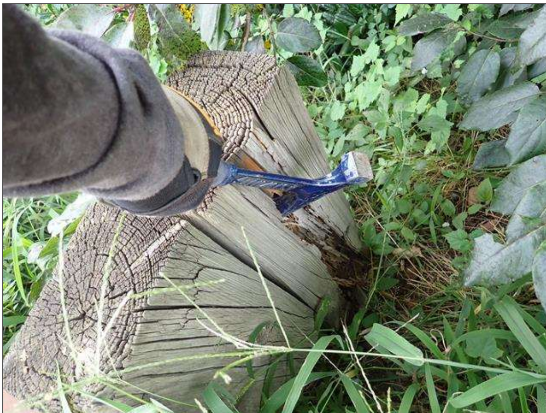
(PAR) southeast guardrail, timber posts 7, 12 and 14, decay/section loss (up to full width x full height x full depth)
