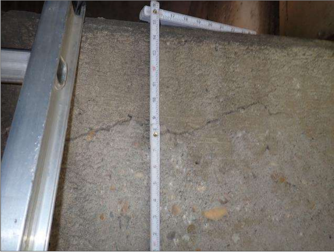
Bent 2 Cap 1: along the length of the cap, near top, longitudinal cracks (up to 1/16 inch x 8 foot) at random
