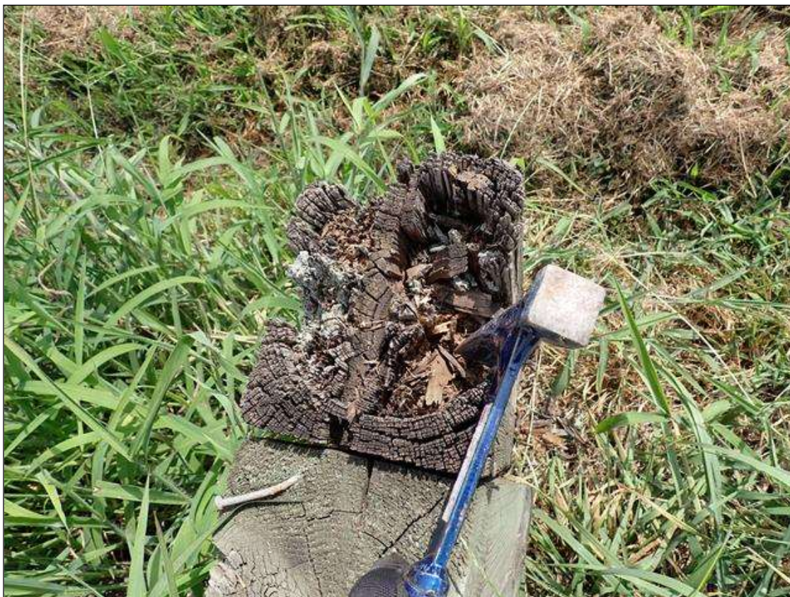
(PAR) southeast guardrail, timber posts 7, 12 and 14, decay/section loss (up to full width x full height x full depth)
