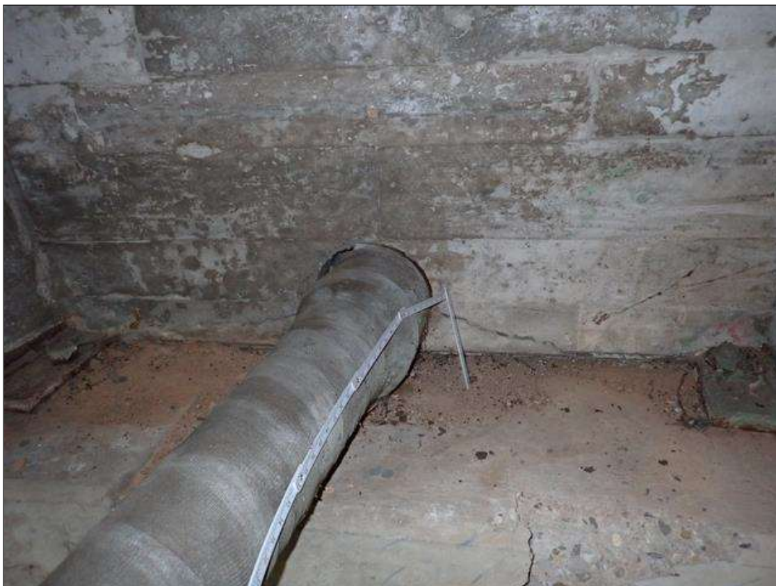
End Bent 2 Abutment: at bay 1 utility penetration, delamination (4 foot x 4 inch) with cracks (up to 1/4 inch)
