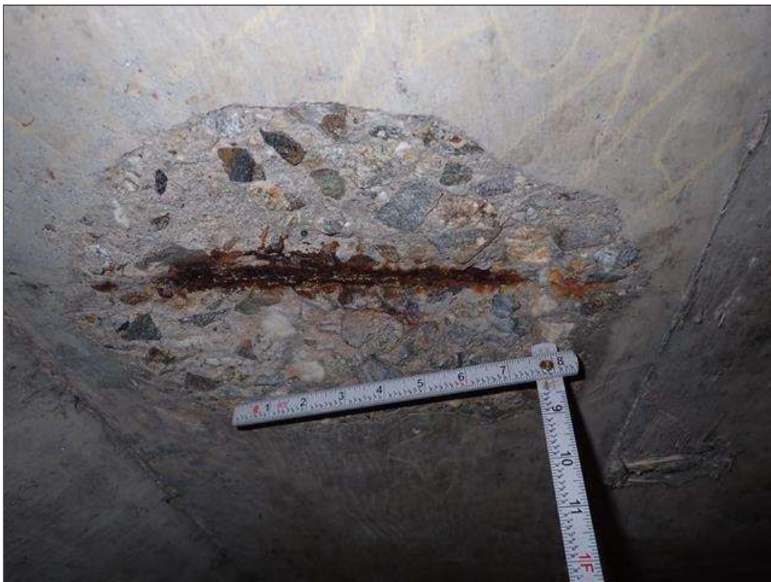
Span 4 Deck: (PAR) under bay 1 at 6 foot from end bent 2, spall [10 inch x 11 inch x up to 1 inch deep] with exposed rusted reinforcing [loss up to 1/16 inch]
