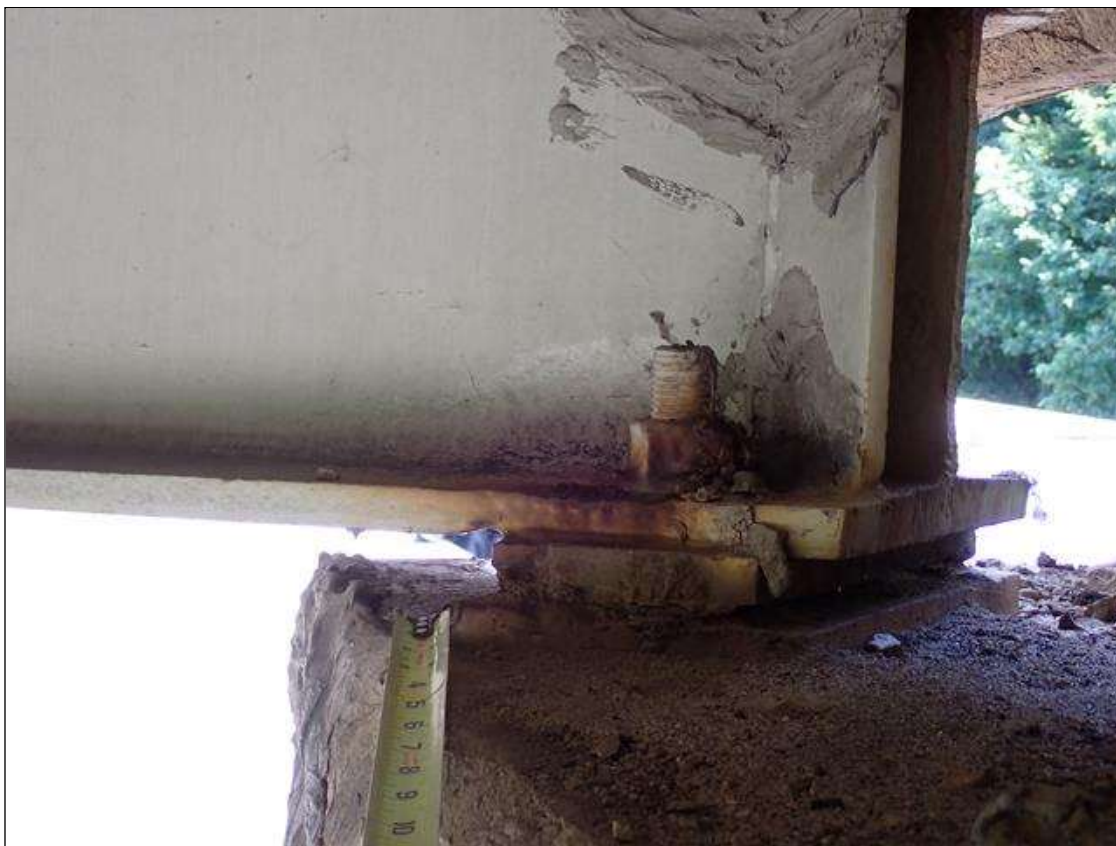
Span 3 Beam 4: at bent 2, painted over section loss: web adjacent to diaphragm (9/16 inch average remaining x 8 inch x 2 inch); lower web (9/16 inch average remaining x 15 inch x 3 inches); bottom flange (1 inch average remaining x 3 inches) with corrosion reinitiated
