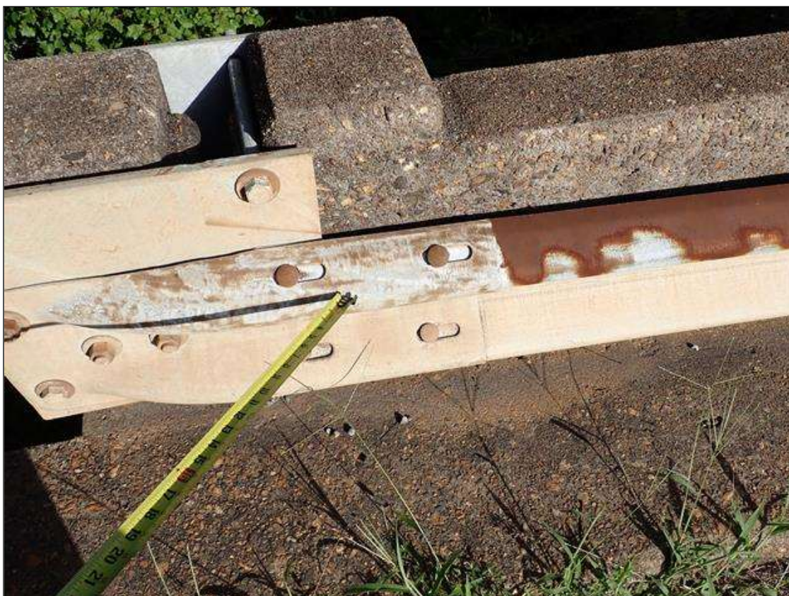
(PAR) northwest guardrail attachment, improper lap
