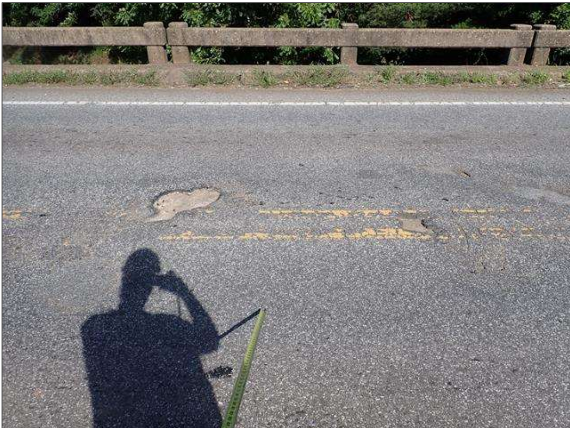
Span 3 Wearing Surface: (PAR) at bent 2, areas of missing asphalt (up to 3 feet x 2 inches) at random; northbound lane, at bent 3, areas of missing asphalt (up to 3.5 feet x 2 feet)
