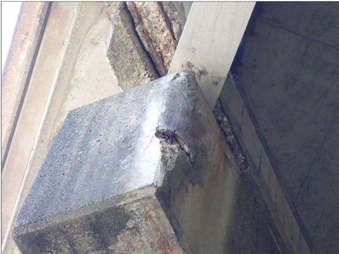
Bent 1 Cap 1: southwest corner, failed patch (full height x 18 inch x up to 2 inches deep) with exposed rusted rebar
