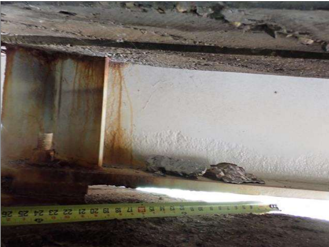
Span 2 Beam 3: at bent 1, painted over section loss: web adjacent to diaphragm (5/8 inch average remaining x 10 inch x 2 inch); lower web (9/16 inch average remaining x 7 feet x 4 inch) with corrosion reinitiated; bottom flange, rust scale
