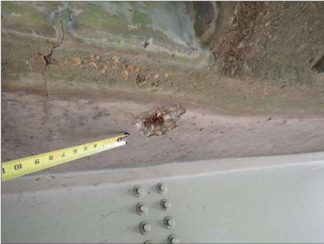
Span 1 Deck: (PAR) left and right overhangs, near end bent 1, spalls (up to 6 inch x 4 inch x 1 inch deep) with exposed rusted rebar
