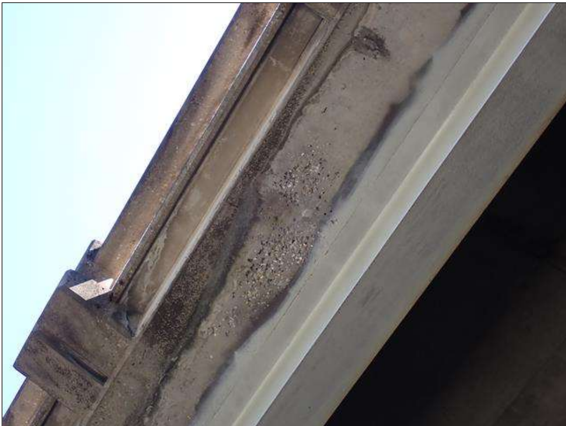
Span 2 Deck: throughout underside of deck, areas of poor consolidation (up to 1/2 inch deep) at random
