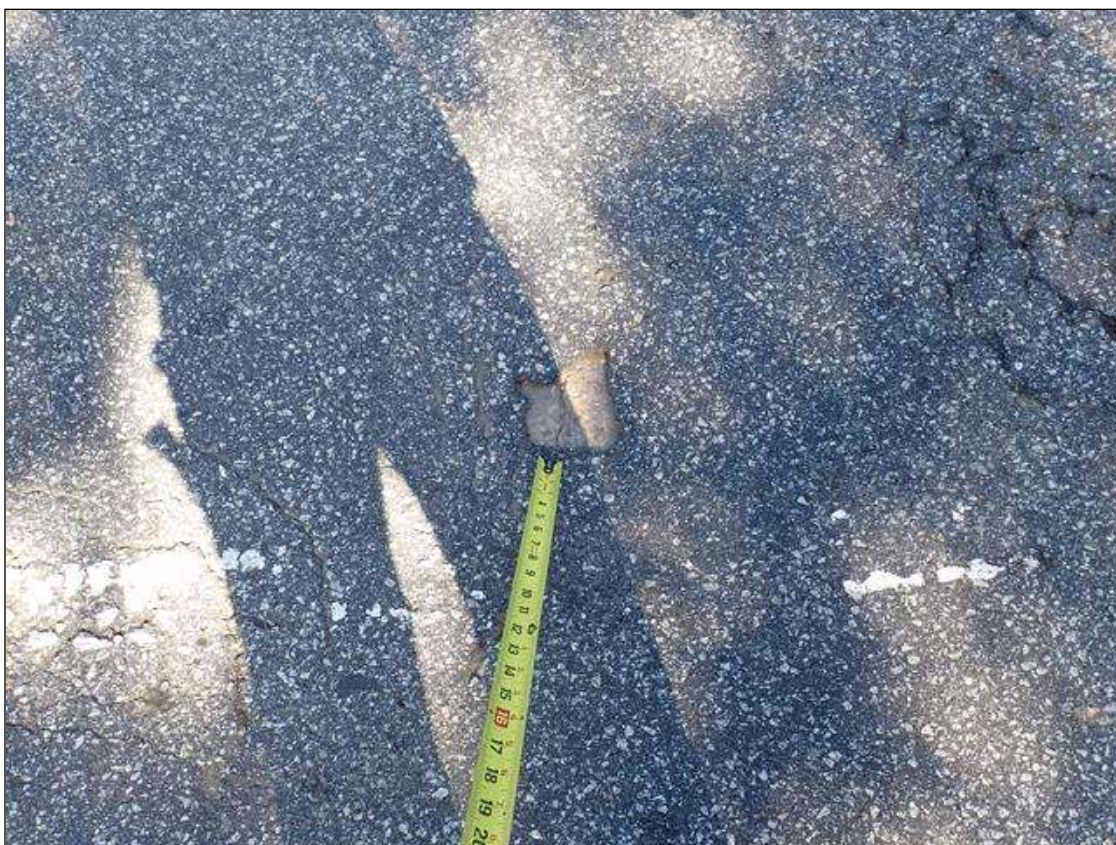
Span 4 Deck: top of deck, northbound lane, near end bent 2, transverse crack (up to 1/32 inch) at area of missing asphalt
