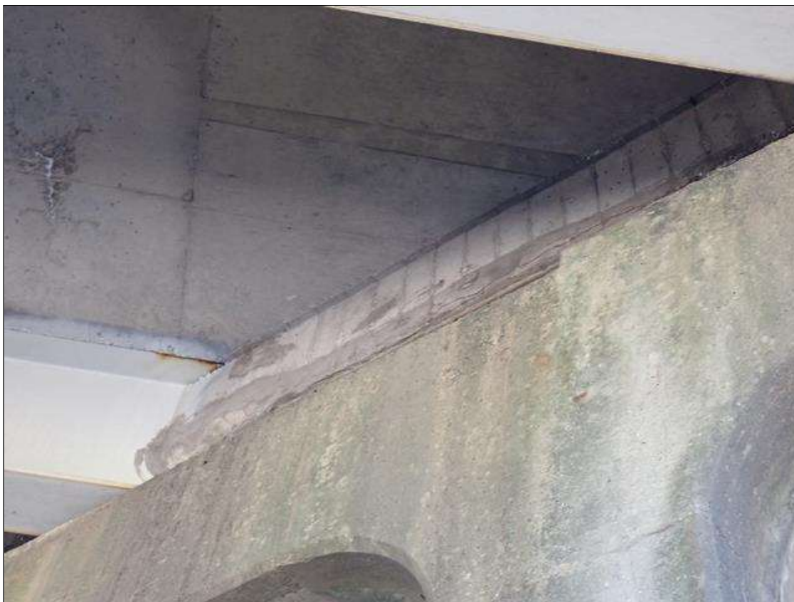
Span 2 Deck: at bent 1, end diaphragms in all bays, and bay 3 diaphragm at bent 2, unsound patches (up to full bay with x 8 inch) with cracks (up to 1/16 inch)
