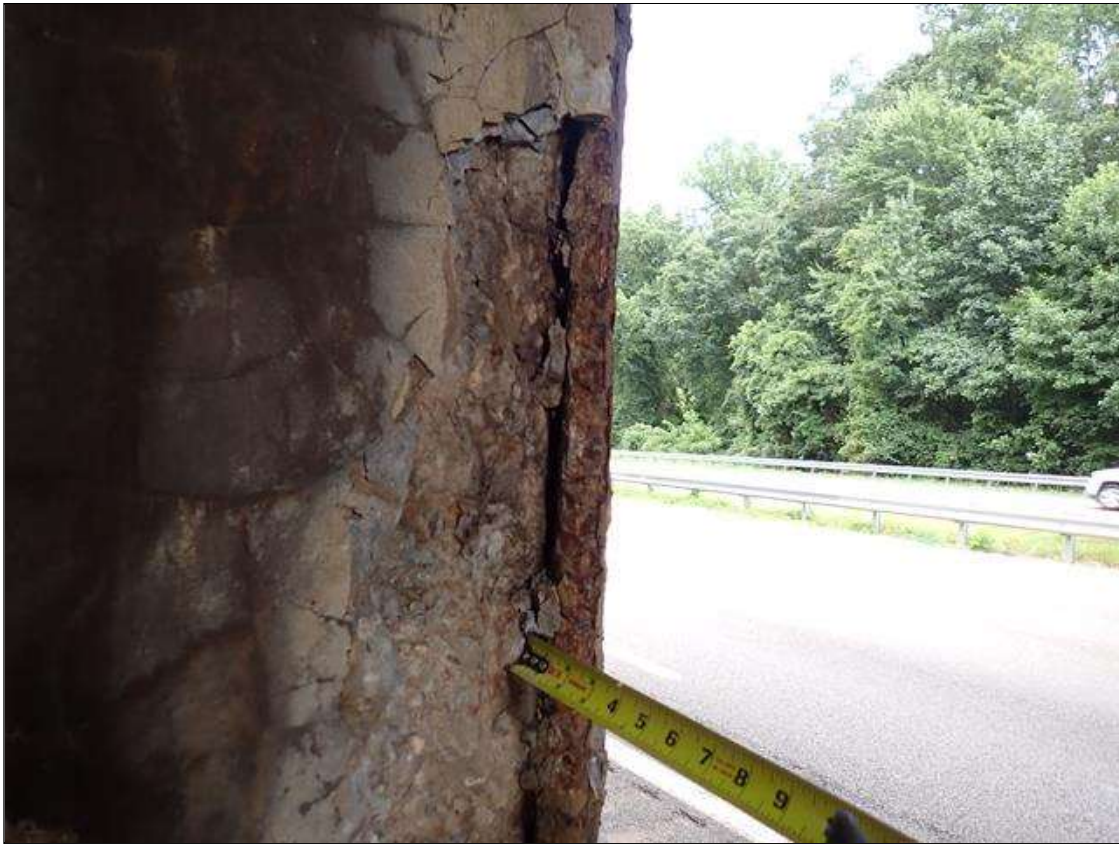
Bent 3 Pile 2: (PAR) at Southwest corner, failed patch, 7 feet high x 22 inches wide x up to 3.5 inches deep with exposed rusted and debonded primary reinforcing
