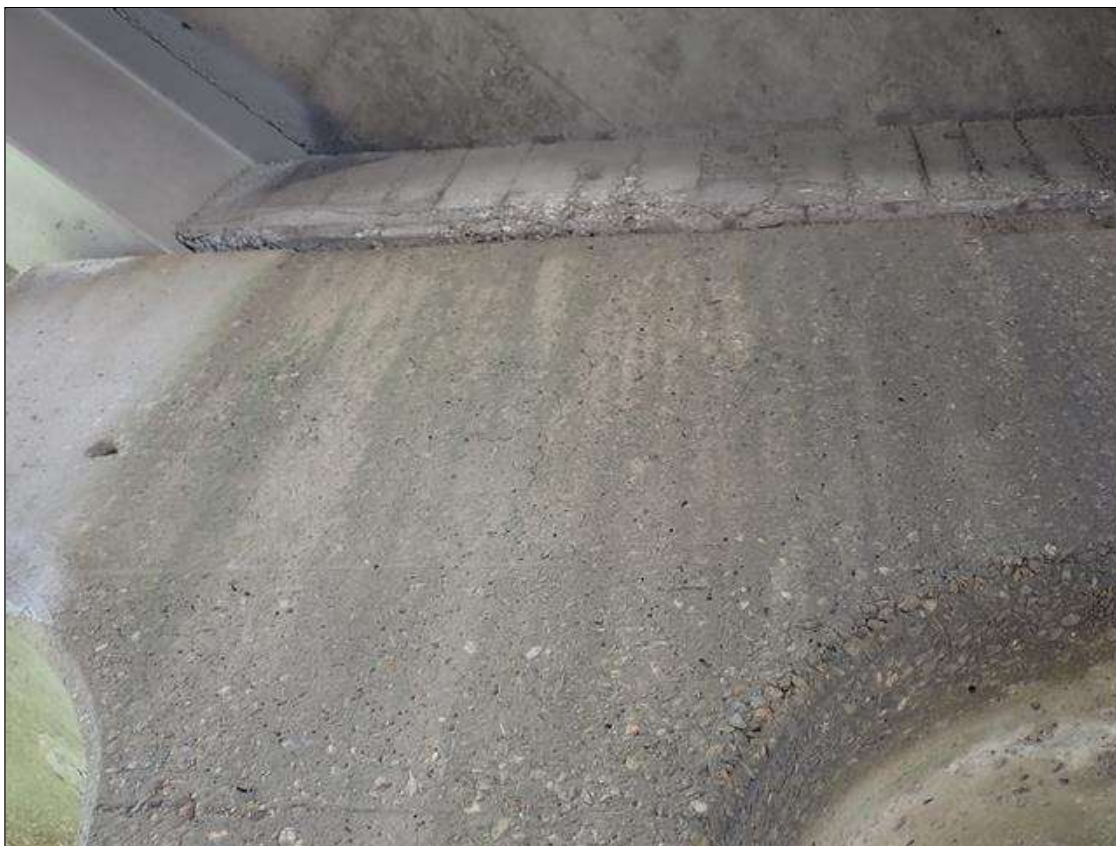
Bent 3 Cap 1: (PAR) UP TO 1/32 INCH MAP CRACKING, SOME WITH EFFLORESCENCE AND RUST STAINS, AT RANDOM THROUGHOUT
