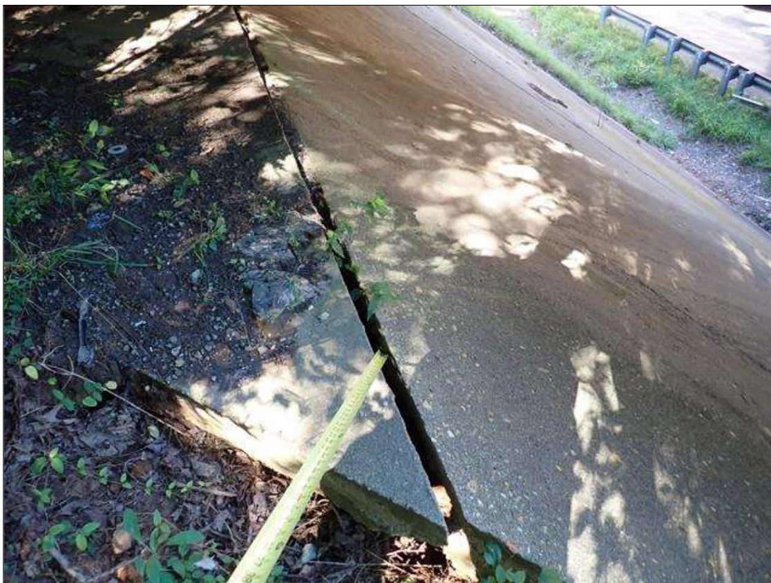
(PAR) end bent 1 slope protection, between slope and end bent berm, gap/settled (up to 2 inches wide x 2 inches high) with undermining (up to 1 foot deep) extending along full width of slope protection
