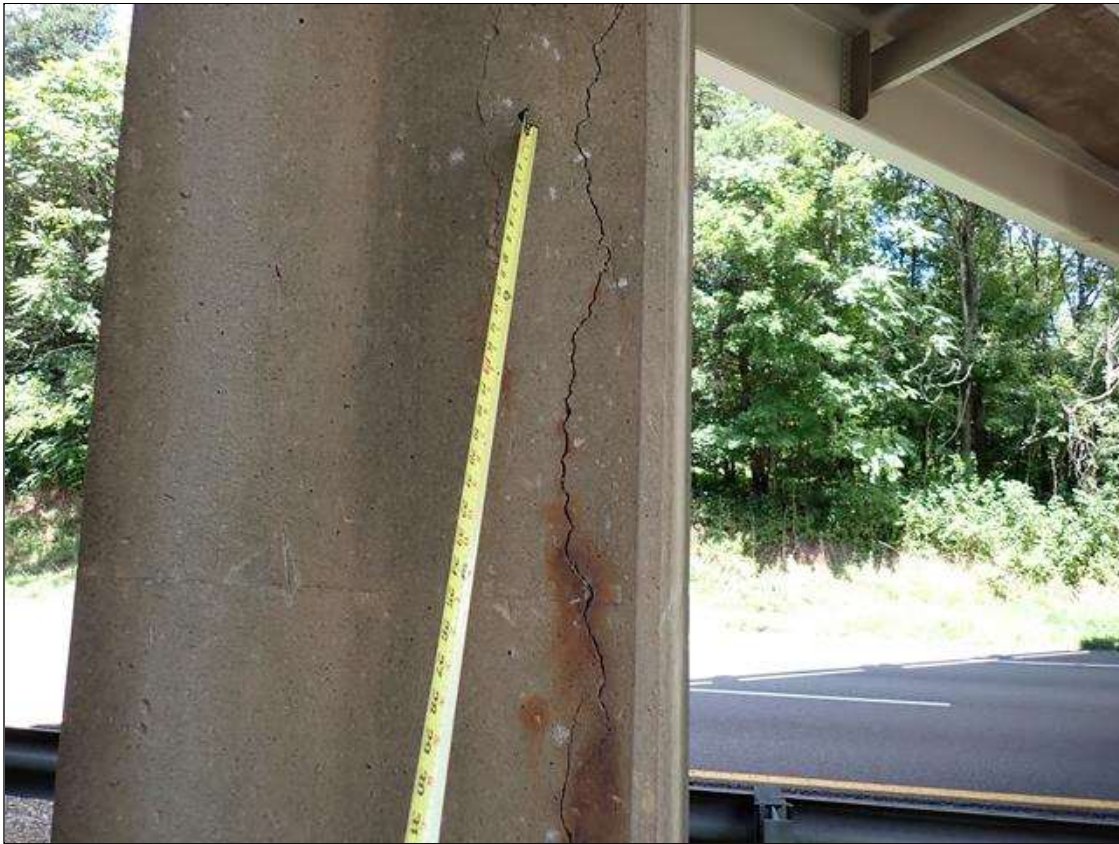
Bent 2 Pile 2: (PAR) at southeast corner, vertical cracks (up to 1/8 inch x full height) with rust stains and adjacent delaminations (up to 4 feet x 6 inch)
