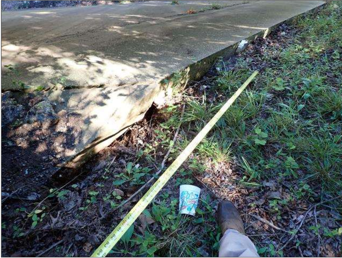
(PAR) east side of span 1, extending from behind southeast wingwall to toe of end bent 1 slope protection, erosion channel (approximately 100 feet long x 3 feet long x 1.5 feet deep) undermining slope protection (up to 1 foot high x 1.5 foot deep)
