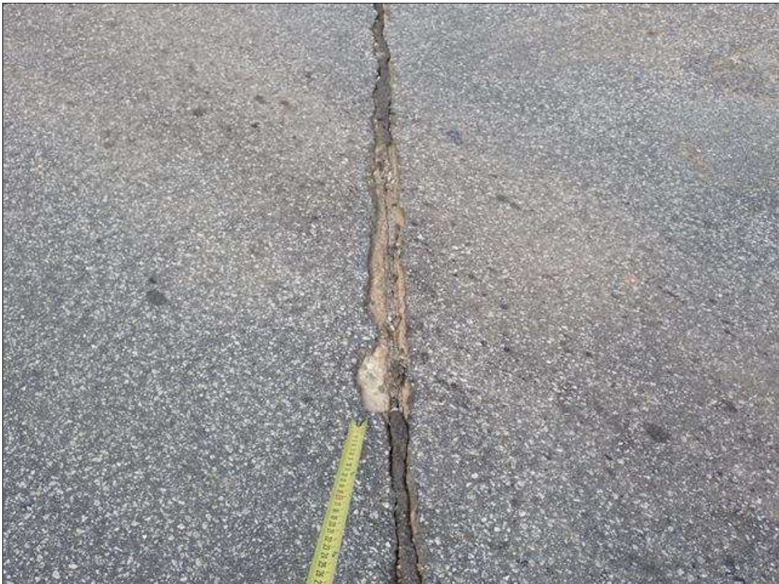
Span 2 Wearing Surface: (PAR) at bent 2, areas of missing asphalt (up to 2 feet x 3 inch) at random
