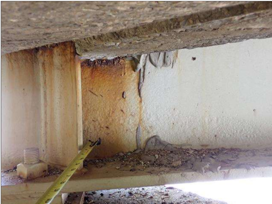
Span 3 Beam 4: at bent 3, web adjacent to diaphragm and lower web, painted over pitting (up to 1/8 inch deep x 2 feet x 9 inches) with corrosion reinitiated
