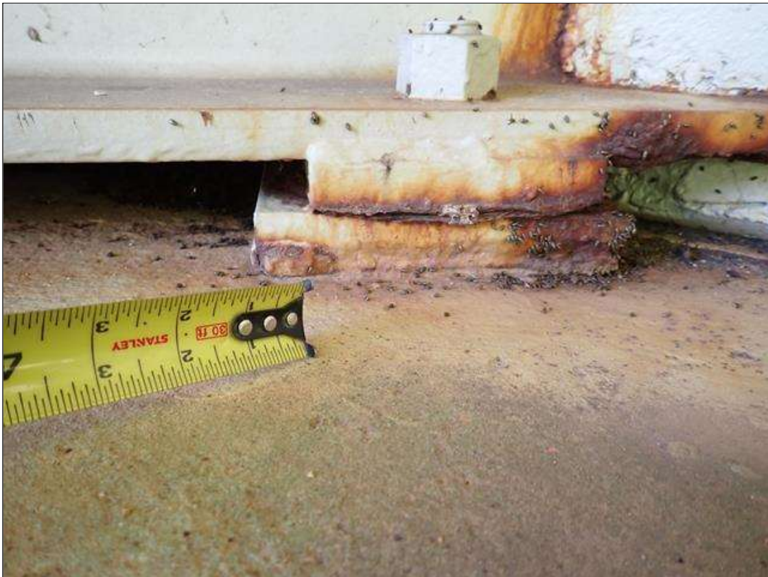
Span 1 Beam 1 - Near Bearing 1: painted over section loss (up to 3/16 inch deep) with corrosion reinitiated
