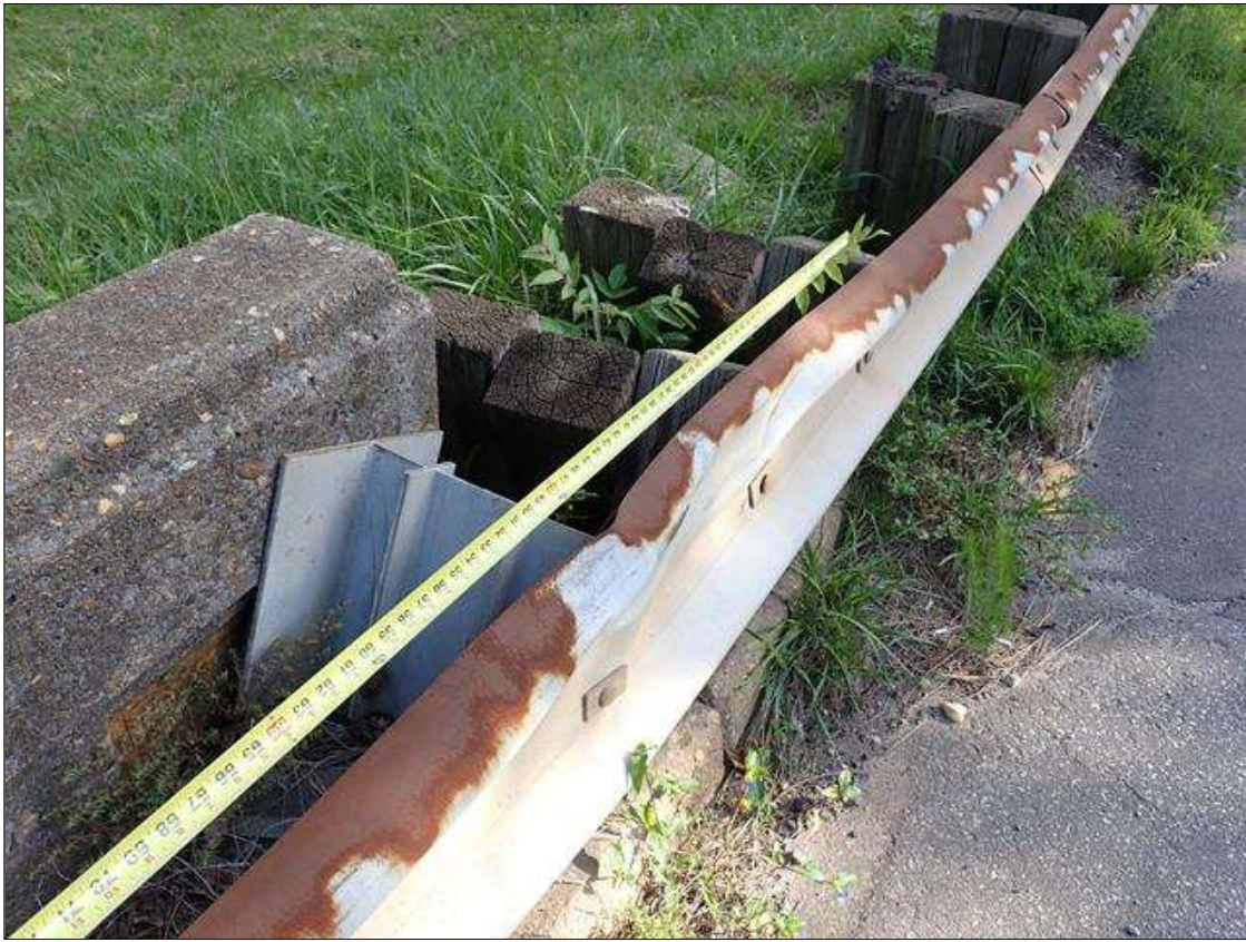
(PAR) northwest guardrail transition, impact damage (5 feet)
