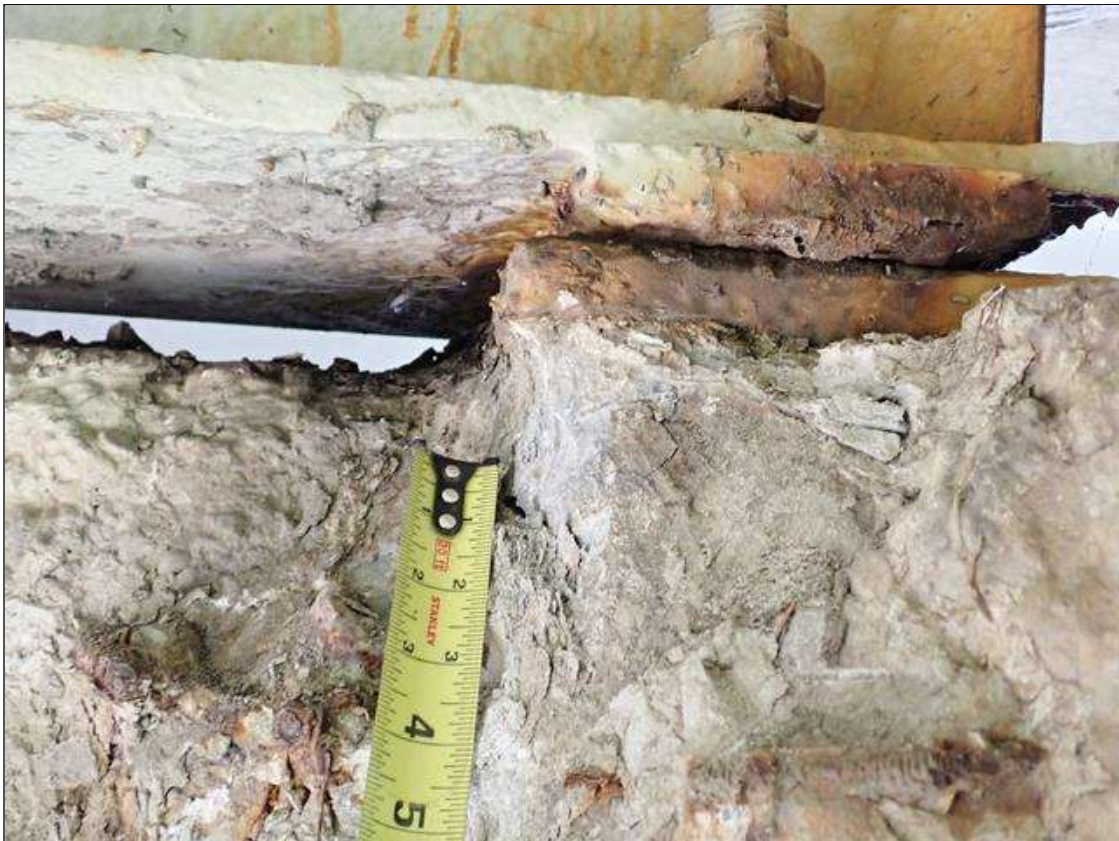
Span 4 Beam 2 - Near Bearing 2: (PAR) northwest corner, loss of bearing (4 inch x 3 inch x up to 1/2 inch deep) due to cap spall
