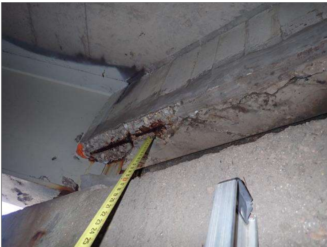
Span 1 Deck: at bent 1, end diaphragm in all bays, spalls/delaminations (up to full bay width x 8 inch x 2 inches deep) with exposed rusted rebar and cracks (up to 1/8 inch)
