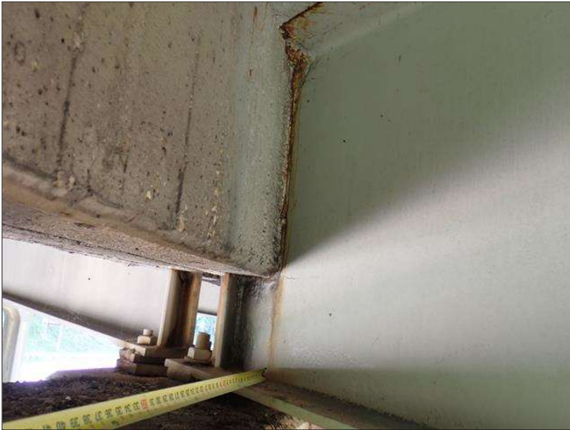
Span 4 Beam 3: (PAR) at bent 3, painted over section loss: web adjacent to diaphragm and upper web (7/16 inch average remaining x 6 inch x 2 foot); lower web (1/2 average remaining x up to 2.5 feet long x 6 inches high); bottom flange (0.77 inch average remaining x 8 inches); top flange, painted over pitting (up to 1/8 inch deep) with corrosion reinitiated
