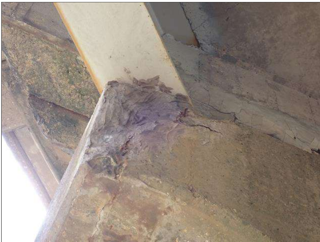
Bent 2 Cap 1: Northeast corner, failed patch with adjacent delamination, 14 inch x 14 inch, and transverse crack, 1/16 inch x full width, on underside of cap
