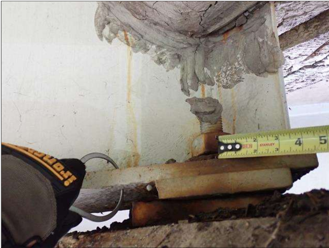
Span 4 Beam 3: (PAR) at bent 3, painted over section loss: web adjacent to diaphragm and upper web (7/16 inch average remaining x 6 inch x 2 foot); lower web (1/2 average remaining x up to 2.5 feet long x 6 inches high); bottom flange (0.77 inch average remaining x 8 inches); top flange, painted over pitting (up to 1/8 inch deep) with corrosion reinitiated
