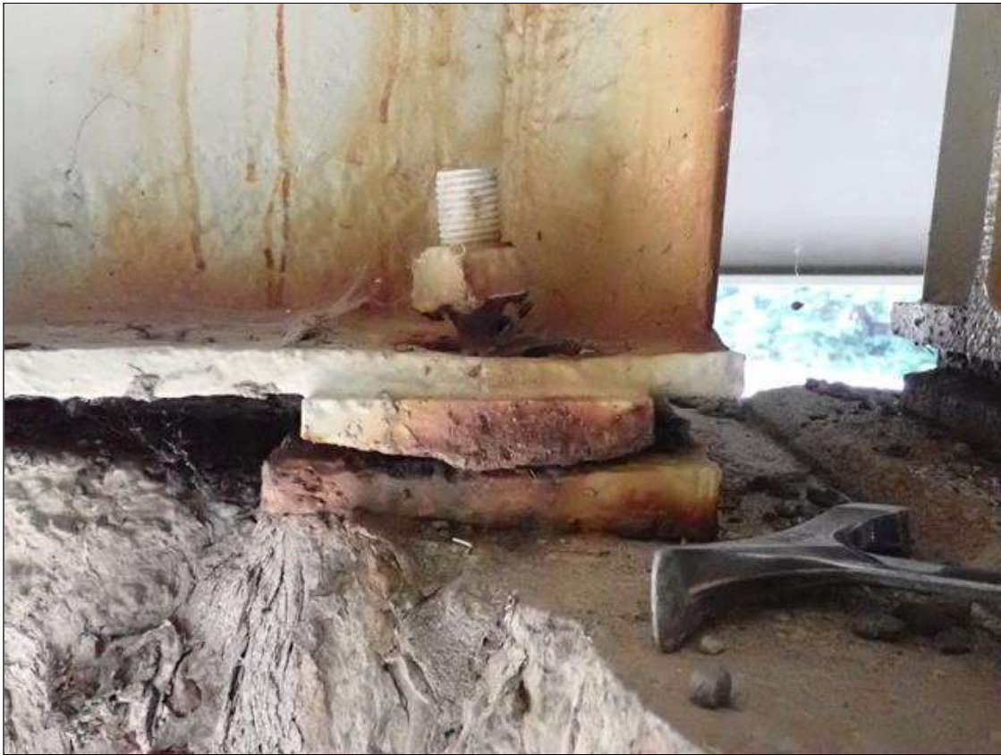
Span 4 Beam 2 - Near Bearing 2: (PAR) painted over section loss (up to 1/8 inch deep); left anchor bolt, approximately 50 percent section loss; pack rust
