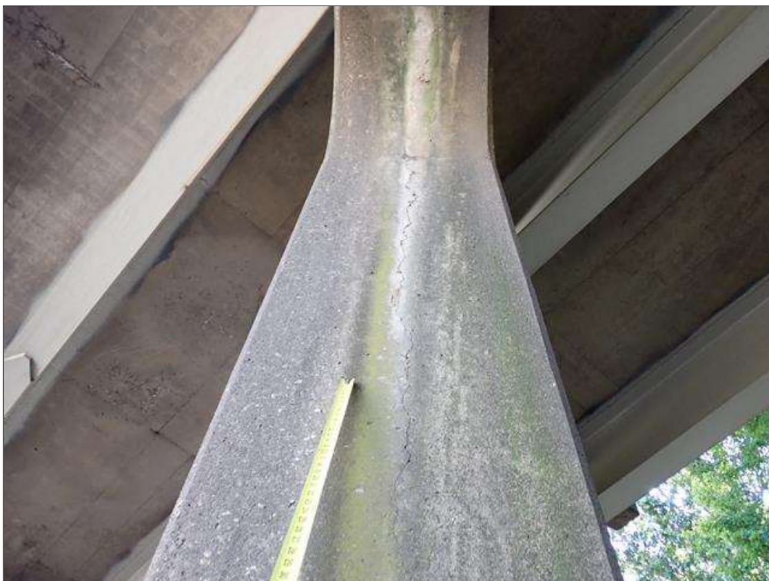
Bent 1 Pile 2: West face at top, vertical crack 9 feet x up to 1/16 inch with adjacent delamination 5 feet x 8 inches
