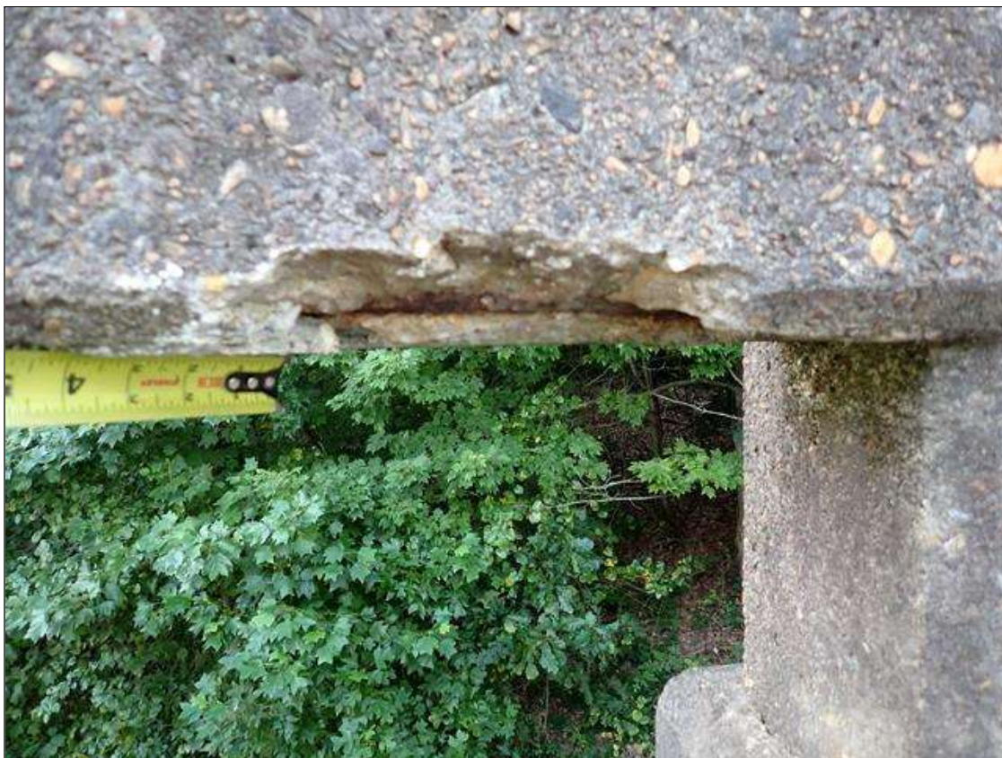
Span 1 Right Bridge Rail: underside of rail section 7, spall (10 inch x 3 inch x 1.5 inch deep) with exposed rusted rebar
