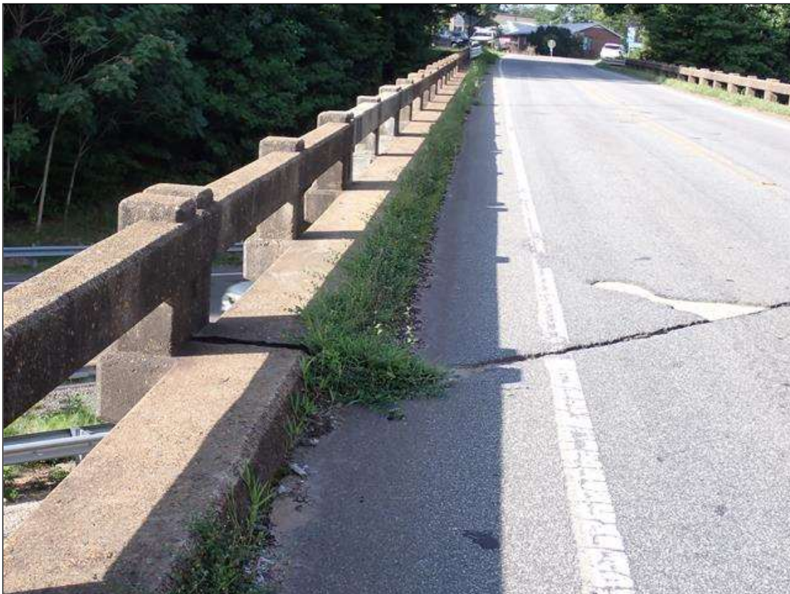
along the curblines, debris accumulation (up to 1.5 feet wide x 3 inches high) with vegetation, obstructing deck drainage
