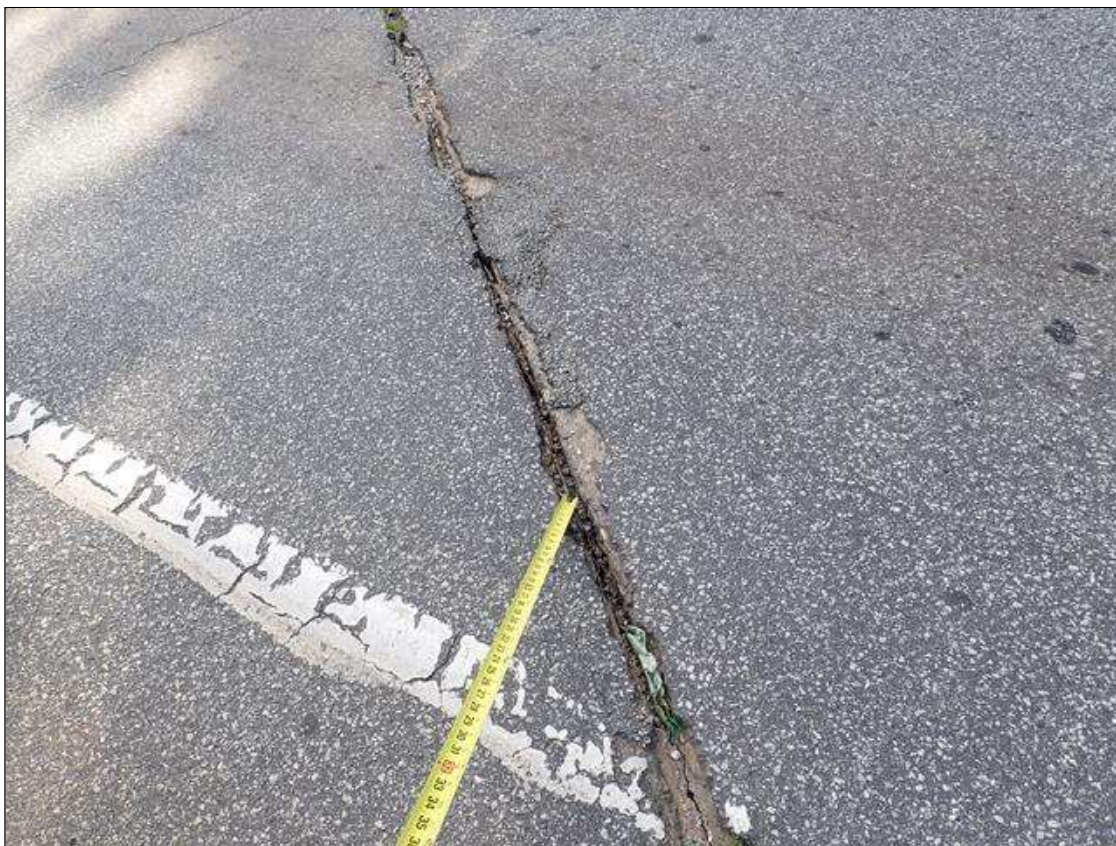
Span 1 Wearing Surface: (PAR) at bent 1, areas of missing asphalt (up to 1 foot x 4 inch)
