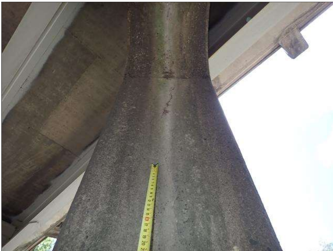
Bent 2 Pile 1: WEST AND EAST FACES, UP TO 1/16 INCH VERTICAL CRACKS AT RANDOM THROUGHOUT.
