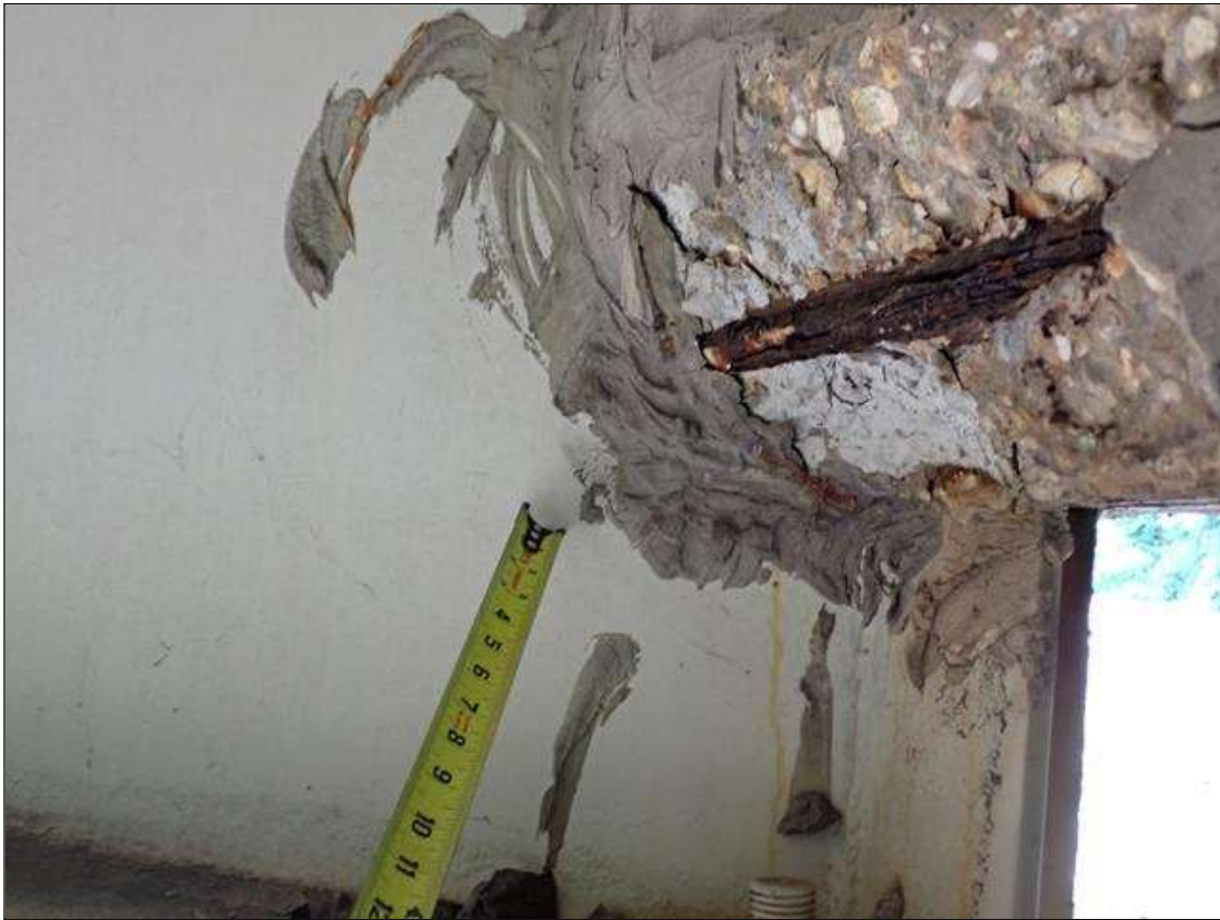
Span 4 Beam 4: at bent 3, web adjacent to diaphragm, painted over section loss (1/2 inch average remaining x 6 inch x 6 inch), partially covered with epoxy
