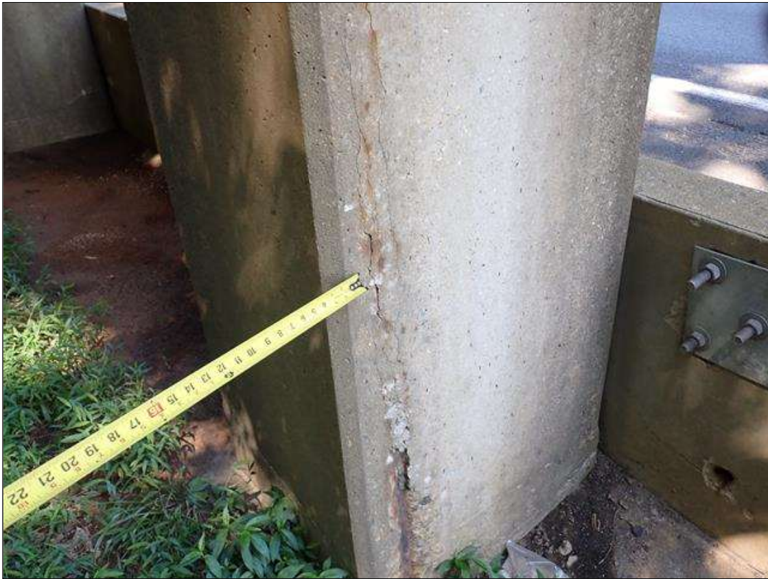
Bent 1 Pile 3: (PAR) southeast and northeast corners, vertical cracks (up to 1/16 inch x 5.5 feet) with rust stains, and adjacent delaminations (up to 4 feet x 6 inch); southeast corner, at ground, spall (2 feet x 6 inch x 1.5 inch deep) with exposed rusted primary reinforcement
