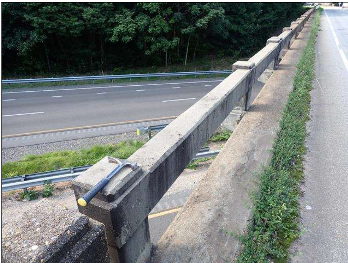
Span 3 Right Bridge Rail: 26 FOOT CONCRETE BRIDGE RAIL REPAIR NEAR MIDSPAN.
