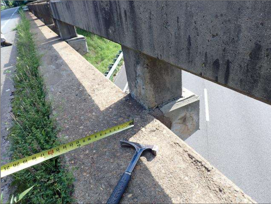
Span 3 Right Bridge Rail: (PAR) within patched area over left and right travel lanes of I-40, area of delamination with cracking (up to 1/16 inch), could possibly fall into traffic below
