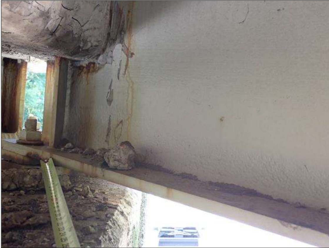
Span 3 Beam 1: at bent 2, web adjacent to diaphragm, painted over section loss (9/16 inch average remaining x 8 inch x 3 inch); lower web, painted over pitting (up to 1/8 inch deep x 7 feet x up to 4 inch) with corrosion reinitiated; bottom flange, rust scale
