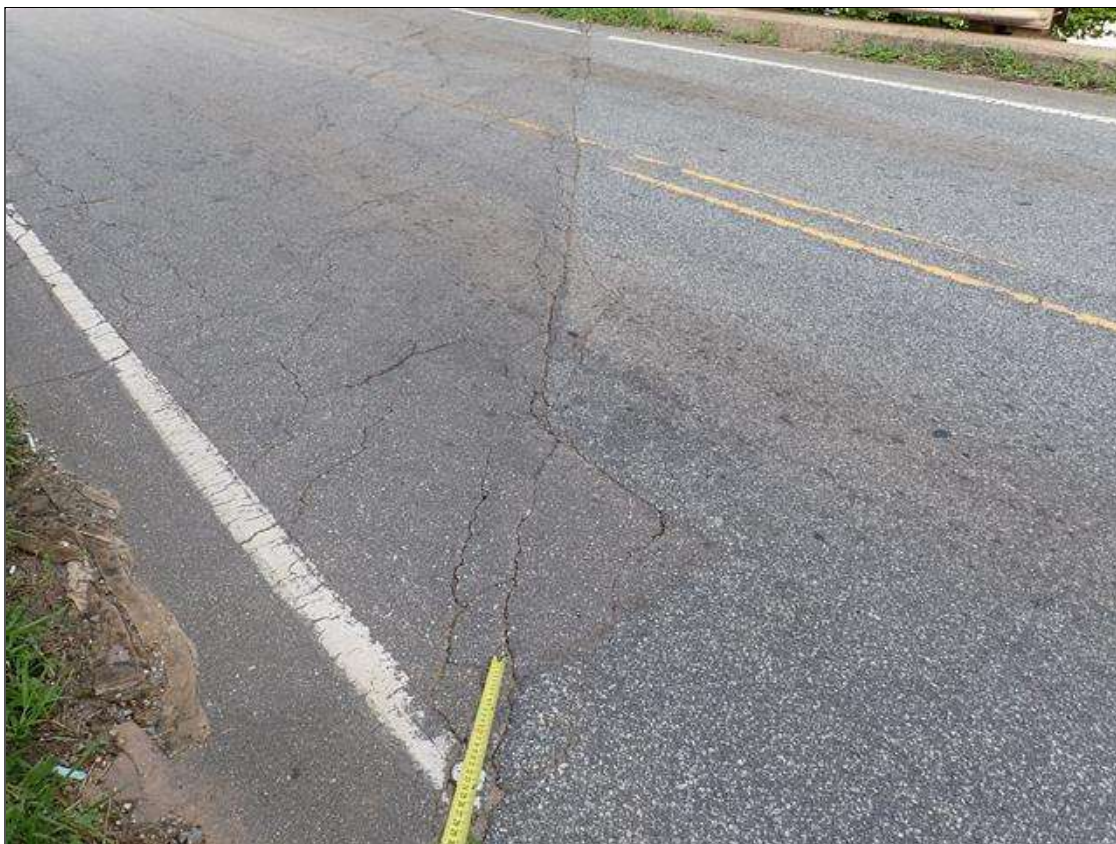
Span 1 Wearing Surface: over end bent 1, transverse cracks, full width x up to 1/2 inch
