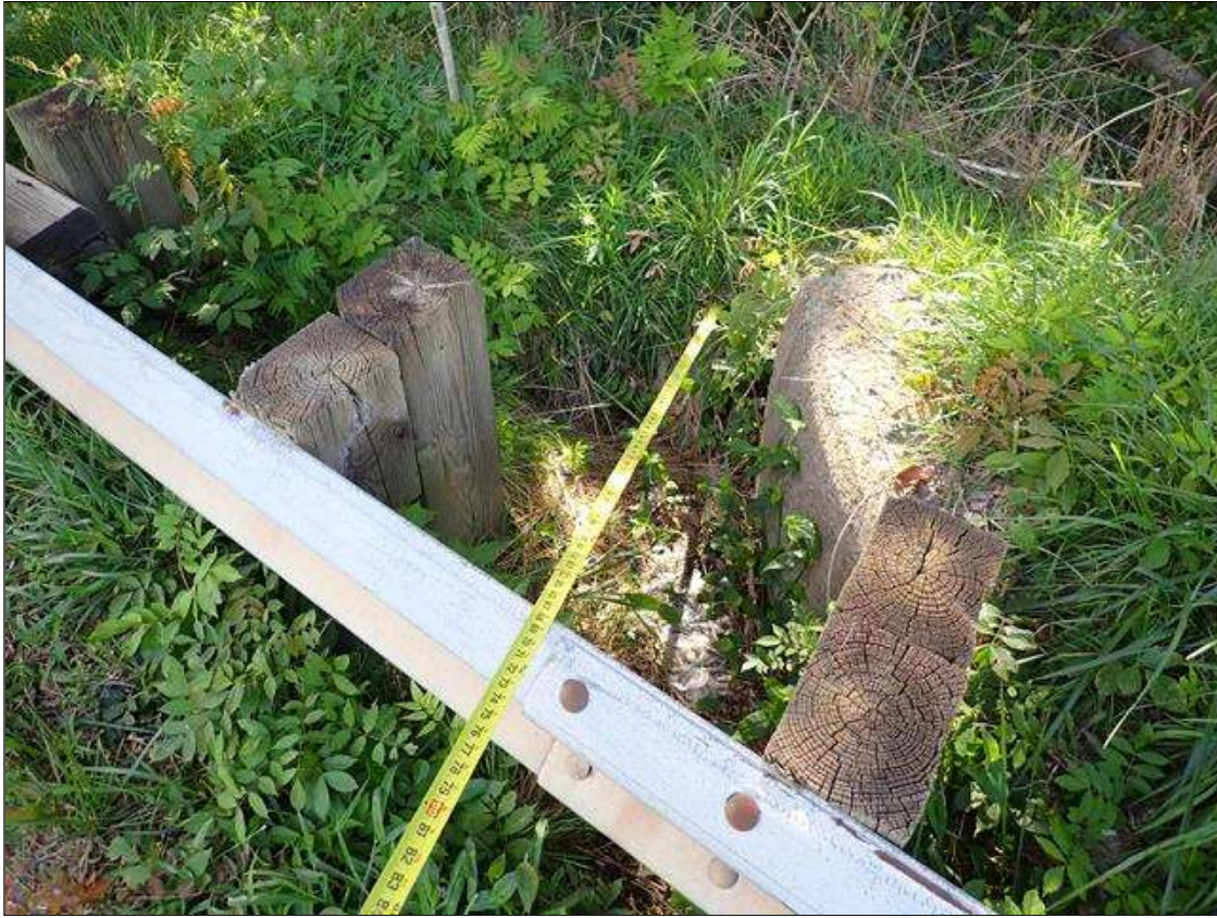
behind northeast approach curb, area of erosion (7 feet x 4 feet x 1.5 feet deep)
