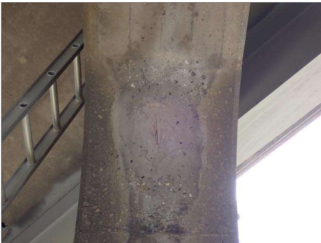
Bent 2 Cap 1: (PAR) underside of cap, adjacent to column 3, patched area (2 feet x 18 inch) with cracks (up to 1/32 inch) and rust stains
