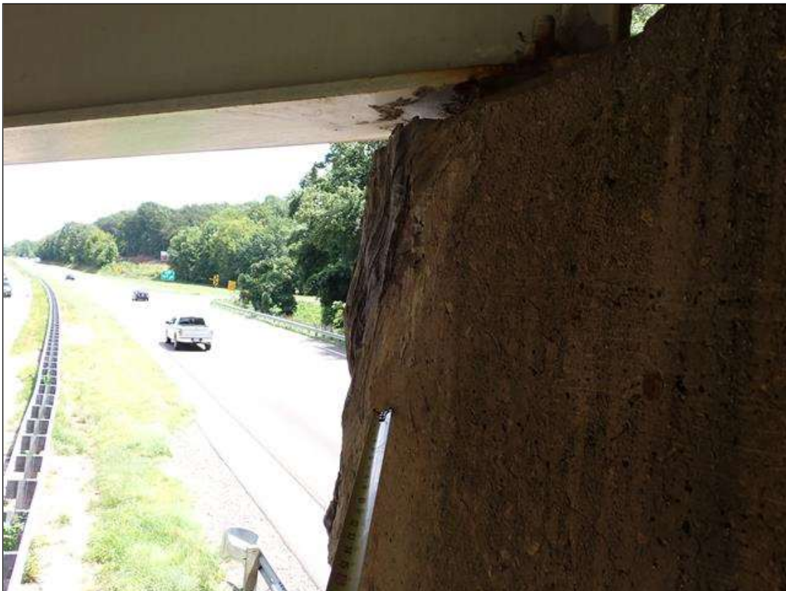
Bent 2 Cap 1: Northeast corner, failed patch with adjacent delamination, 14 inch x 14 inch, and transverse crack, 1/16 inch x full width, on underside of cap
