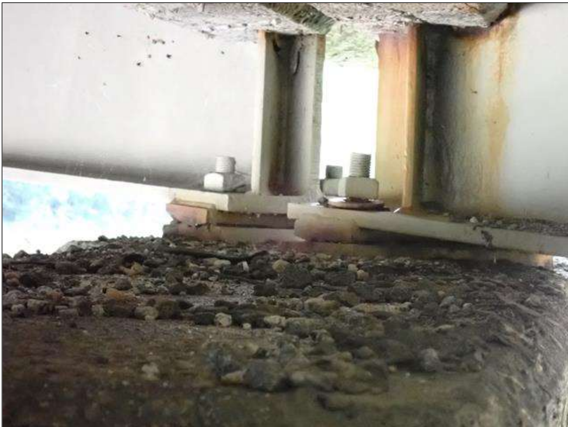
interior bearing assembly
