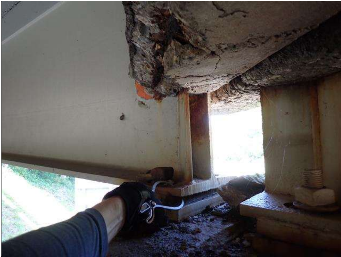
Span 1 Beam 1: at bent 1, painted over section loss: web adjacent to diaphragm (9/16 inch average remaining x 3 inch x 4 inch); bottom flange (0.85 inch x 6 inches) with corrosion reinitiated
