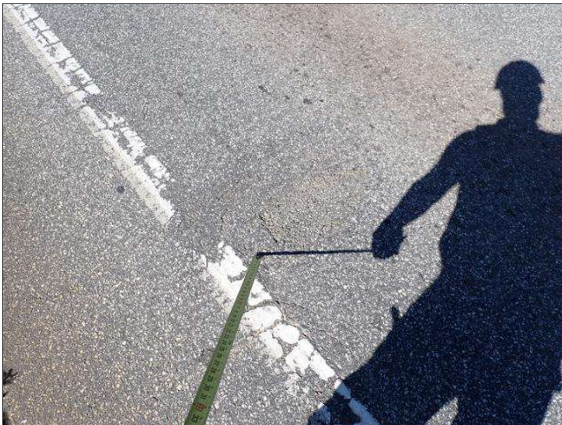
Span 4 Wearing Surface: 2023 previously repaired, previously noted as: midspan Northbound lane near shoulder, pothole, 3 inch x 4 inch x full depth
