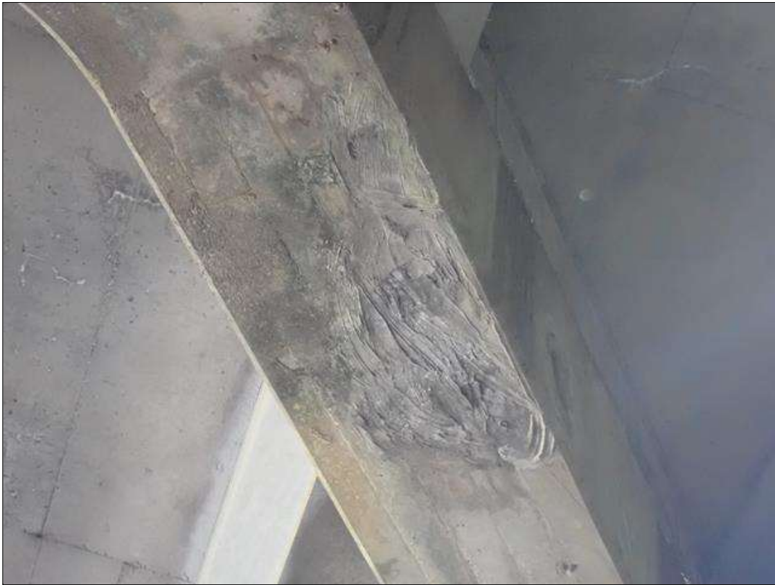
Bent 1 Cap 1: SOUTH FACE AND BOTTOM OF WEST END, AND BETWEEN COLUMNS 2 AND 3. HAS PATCHED AREAS UP TO 3 FEET X 15 INCHES WITH SOME HAIRLINE CRACKS AND EFFLORESCENCE VISIBLE.
