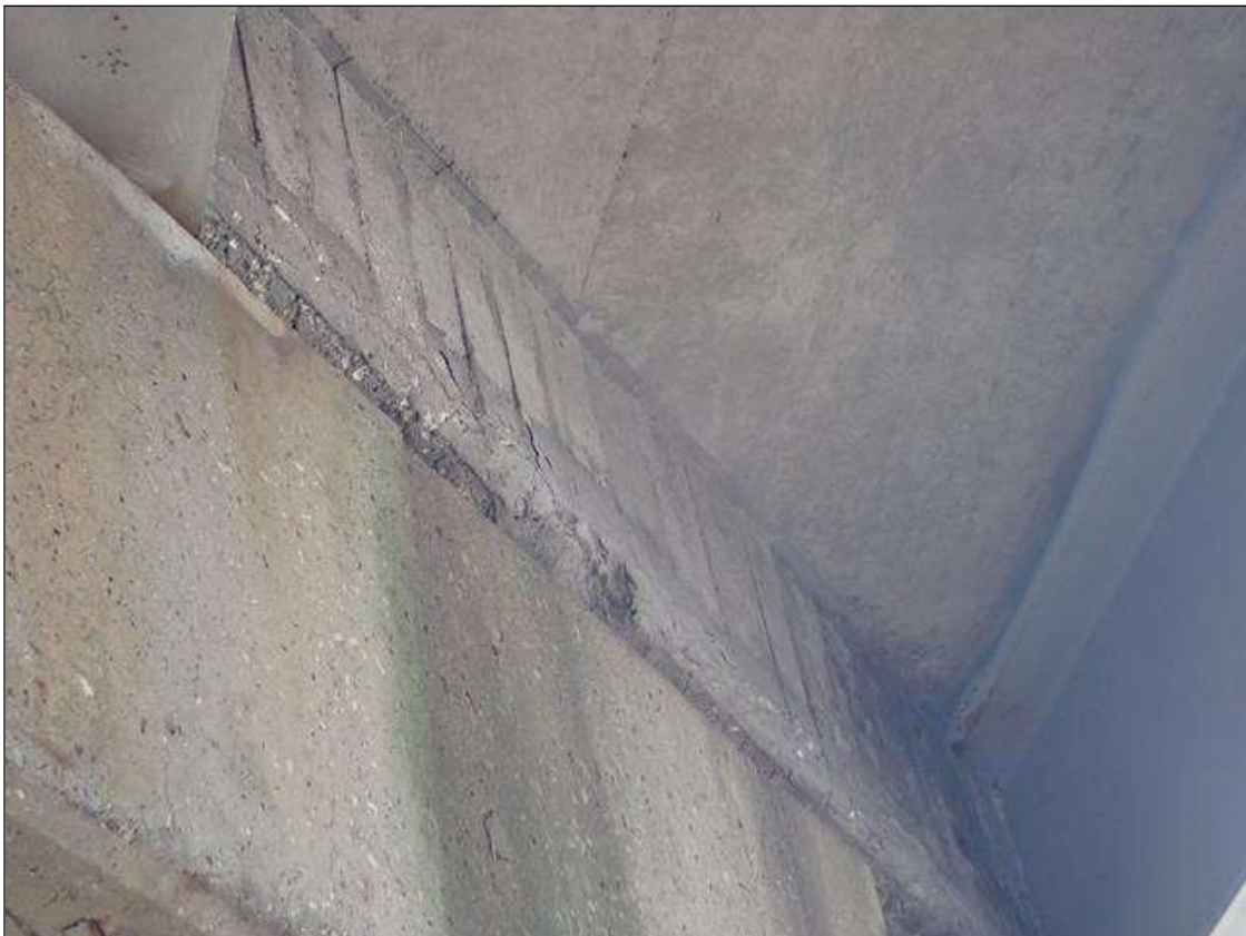
Span 3 Deck: at bents 2 and 3, end diaphragms in all bays, unsound patches/delaminations/spalls (up to full bay width x 8 inch x 1.5 inch deep), some with exposed rusted rebar
