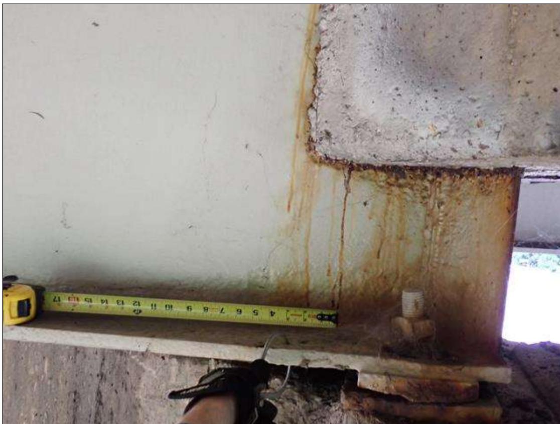
Span 4 Beam 2: (PAR) at bent 3, painted over section loss: web adjacent to diaphragm (7/16 inch average remaining x 7 inch x 2 inch); lower web (1/2 inch average remaining x 4.5 feet x 4 inches); bottom flange (0.71 inch average remaining x 6 inches) with corrosion reinitiated
