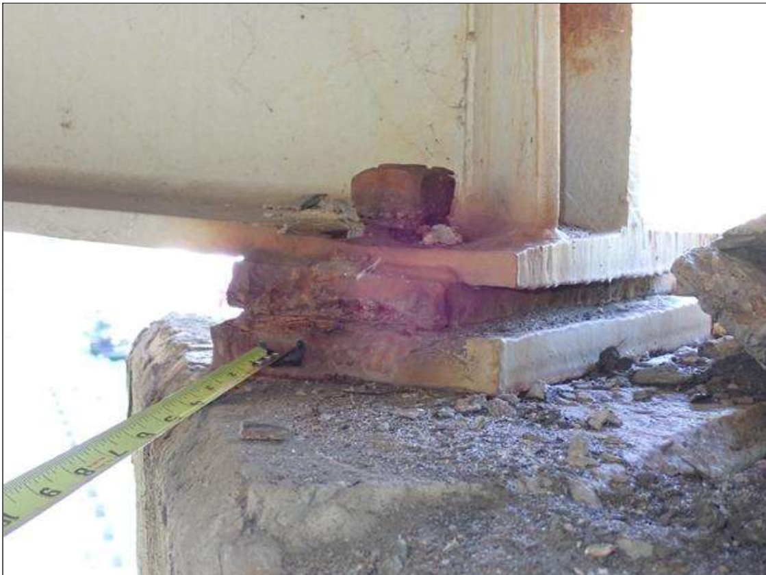
Span 1 Beam 1 - Far Bearing 1: painted over section loss (up to 1/8 inch deep) with corrosion reinitiated; pack rust
