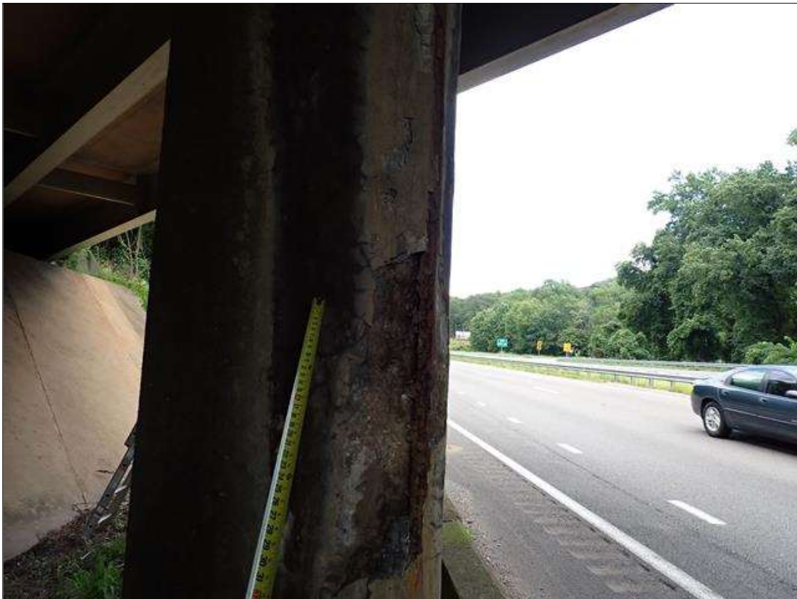
Bent 3 Pile 2: (PAR) at Southwest corner, failed patch, 7 feet high x 22 inches wide x up to 3.5 inches deep with exposed rusted and debonded primary reinforcing
