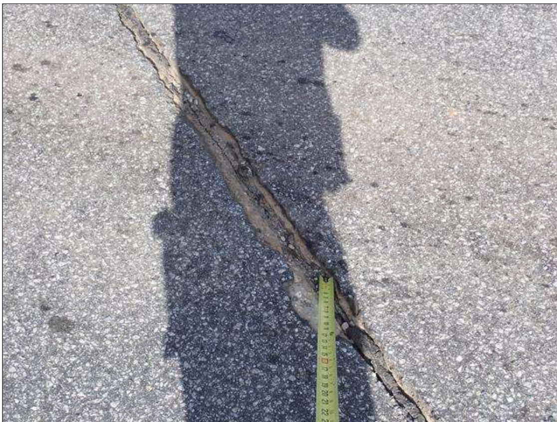
Span 3 Wearing Surface: (PAR) at bent 2, areas of missing asphalt (up to 3 feet x 2 inches) at random; northbound lane, at bent 3, areas of missing asphalt (up to 3.5 feet x 2 feet)
