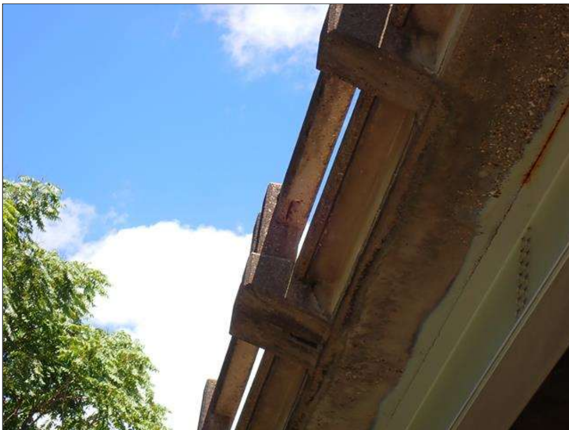
Span 3 Left Bridge Rail: underside of rail, and outriggers, shallow rebar at random
