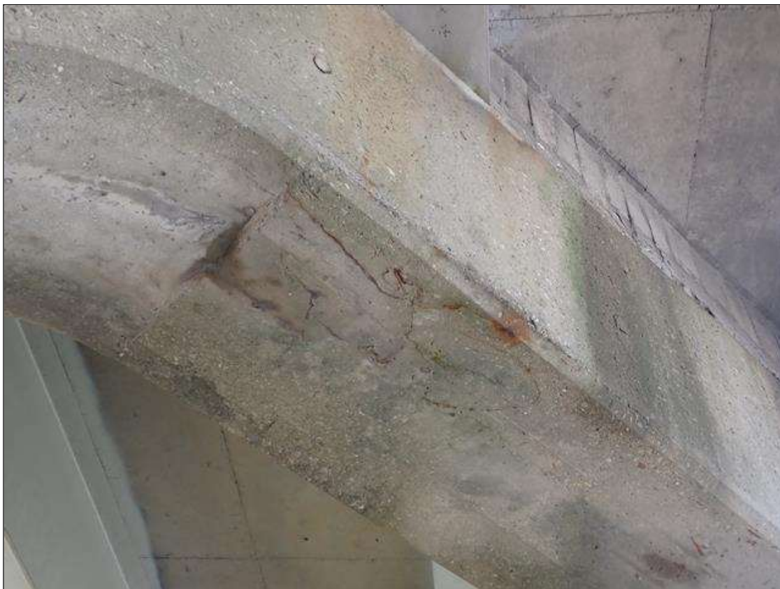
Bent 3 Cap 1: (PAR) UP TO 1/32 INCH MAP CRACKING, SOME WITH EFFLORESCENCE AND RUST STAINS, AT RANDOM THROUGHOUT
