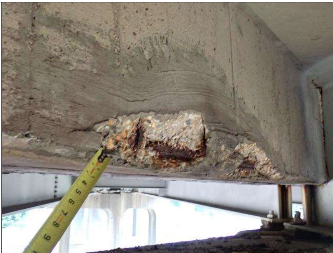
Span 4 Deck: at bent 3, end diaphragms in all bays, failed patches/delaminations/spalls (3.5 feet x 10 inch x 2 inches deep) with exposed rusted rebar
