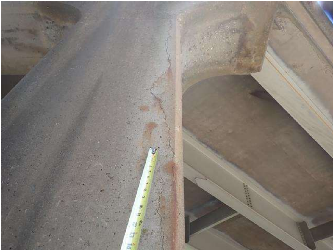
Bent 2 Pile 3: (PAR) UP TO 1/8 INCH VERTICAL CRACKS WITH RUST STAINS AT RANDOM THROUGHOUT with adjacent delaminations up to 6 feet x 1 foot
