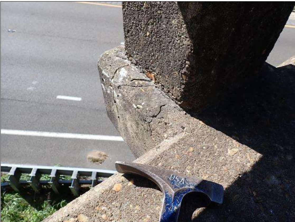
Span 4 Right Bridge Rail: at rail post 2, cracks (up to 1/16 inch wide); adjacent rail section, vertical crack (up to 1/32 inch)
