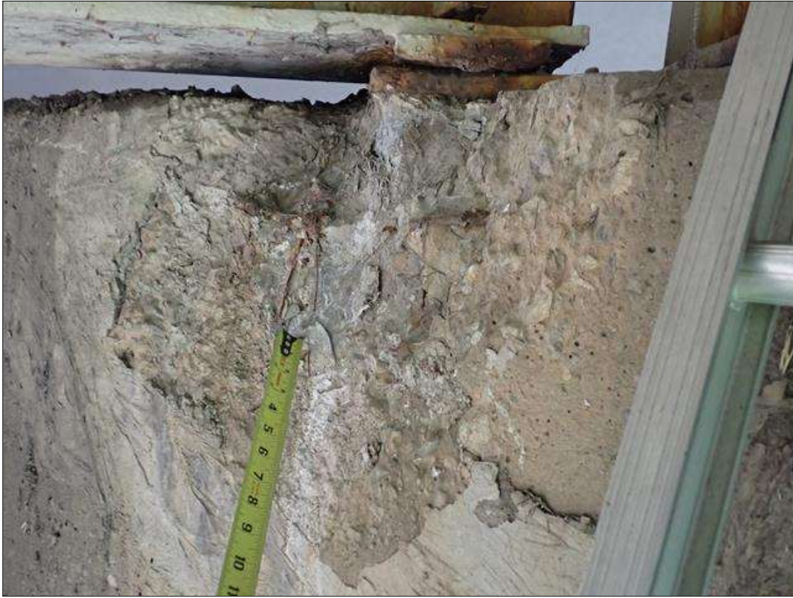
Bent 3 Cap 1: (PAR) 3 FOOT X 18 INCH X 4 INCH DEEP FAILED PATCH/SPALL WITH EXPOSED REINFORCING, CAUSING LOSS OF BEARING, AT PREVIOUSLY PATCHED AREA NORTH FACE BELOW BEAM 2.
