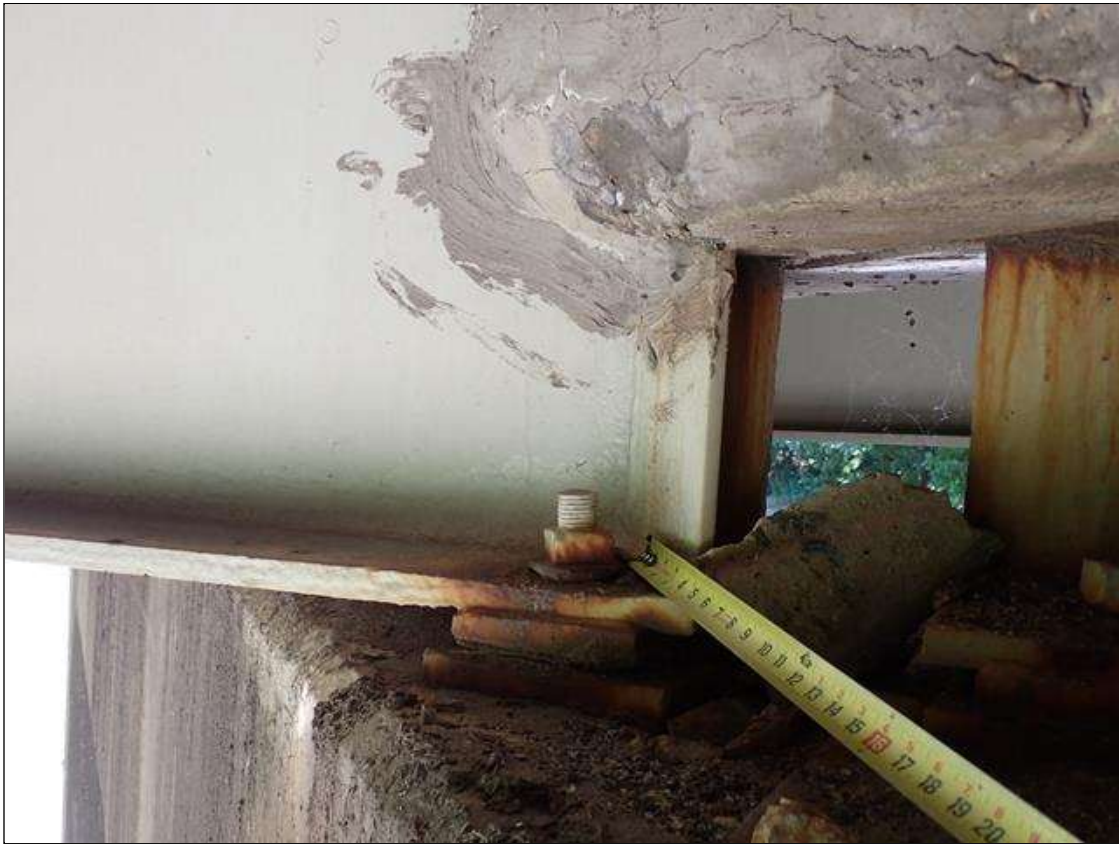
Span 3 Beam 2: at bent 2, painted over section loss: web adjacent to diaphragm (9/16 inch average remaining x 4 inch x 2 inch); lower web (5/8 inch average remaining x 14 inch x 4 inches); bottom flange (1 inch average remaining x 10 inches) with corrosion reinitiated
