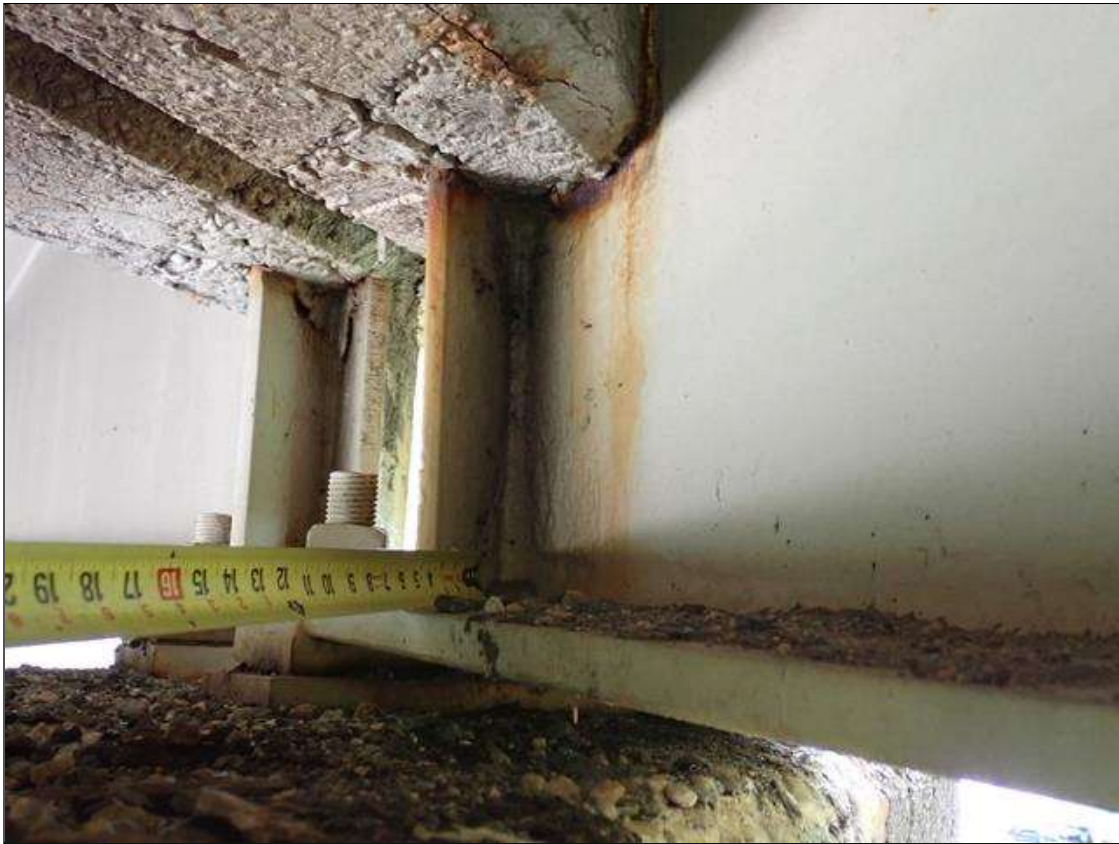
Span 4 Beam 1: at bent 3, painted over section loss: web adjacent to diaphragm (1/2 inch average remaining x 7 inch x 2 inch); lower web (1/2 inch average remaining x 5 inch x 5 inch); bottom flange (0.86 inch average remaining x 1 foot) with corrosion reinitiated
