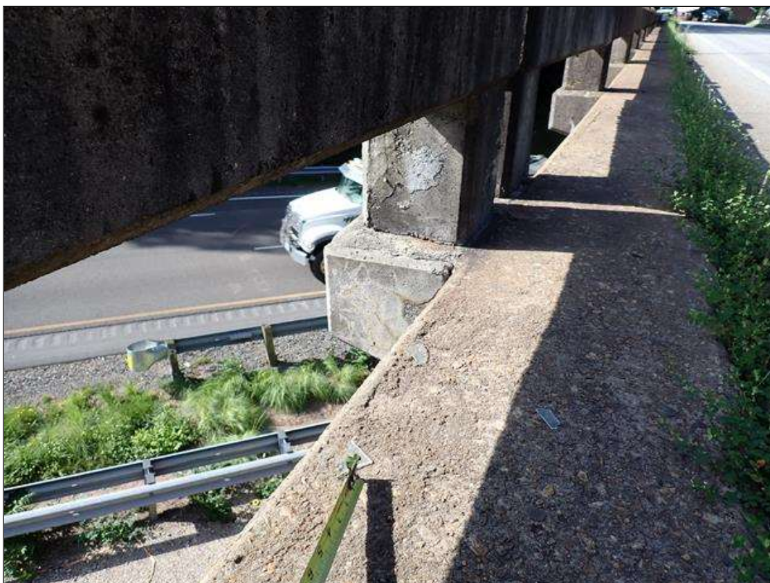
Span 3 Right Bridge Rail: (PAR) within patched area over left and right travel lanes of I-40, area of delamination with cracking (up to 1/16 inch), could possibly fall into traffic below
