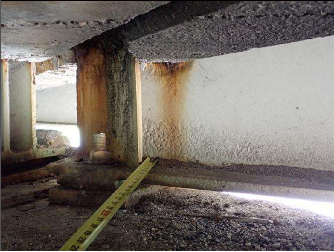
Span 2 Beam 2: at bent 1, painted over section loss: web adjacent to diaphragm (9/16 inch average remaining x 14 inch x 2 inch); lower web (9/16 inch average remaining x 2 feet x 4 inch) with corrosion reinitiated
