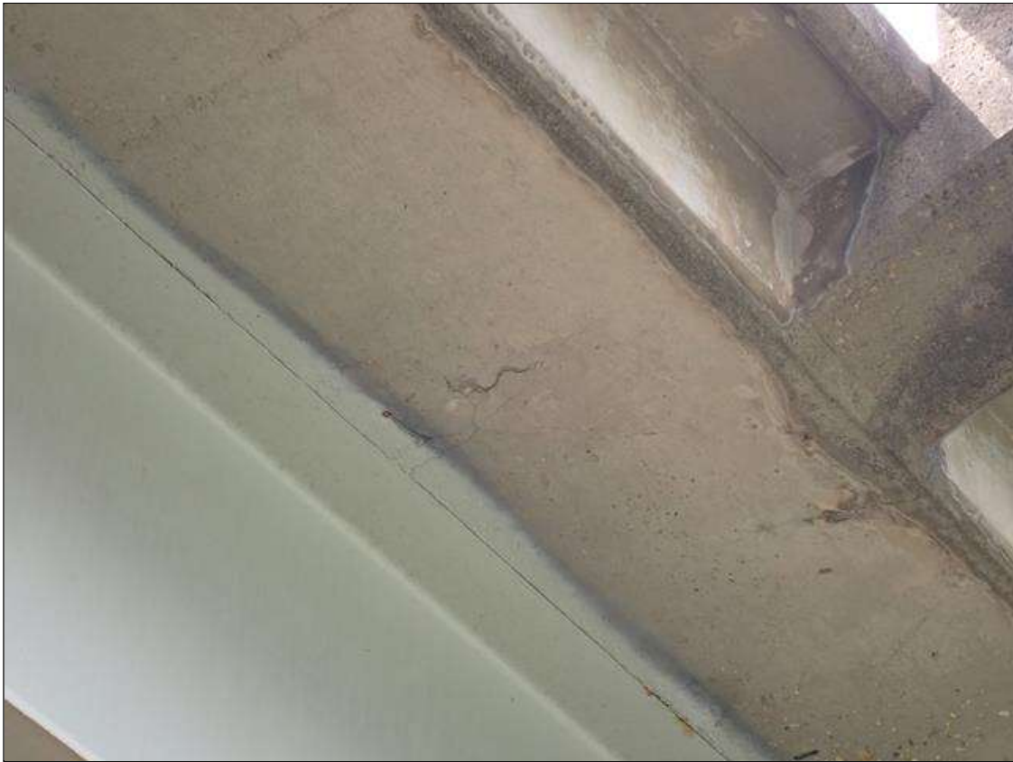
Span 4 Deck: right overhang, near midspan, delamination (10 inch x 6 inch)
