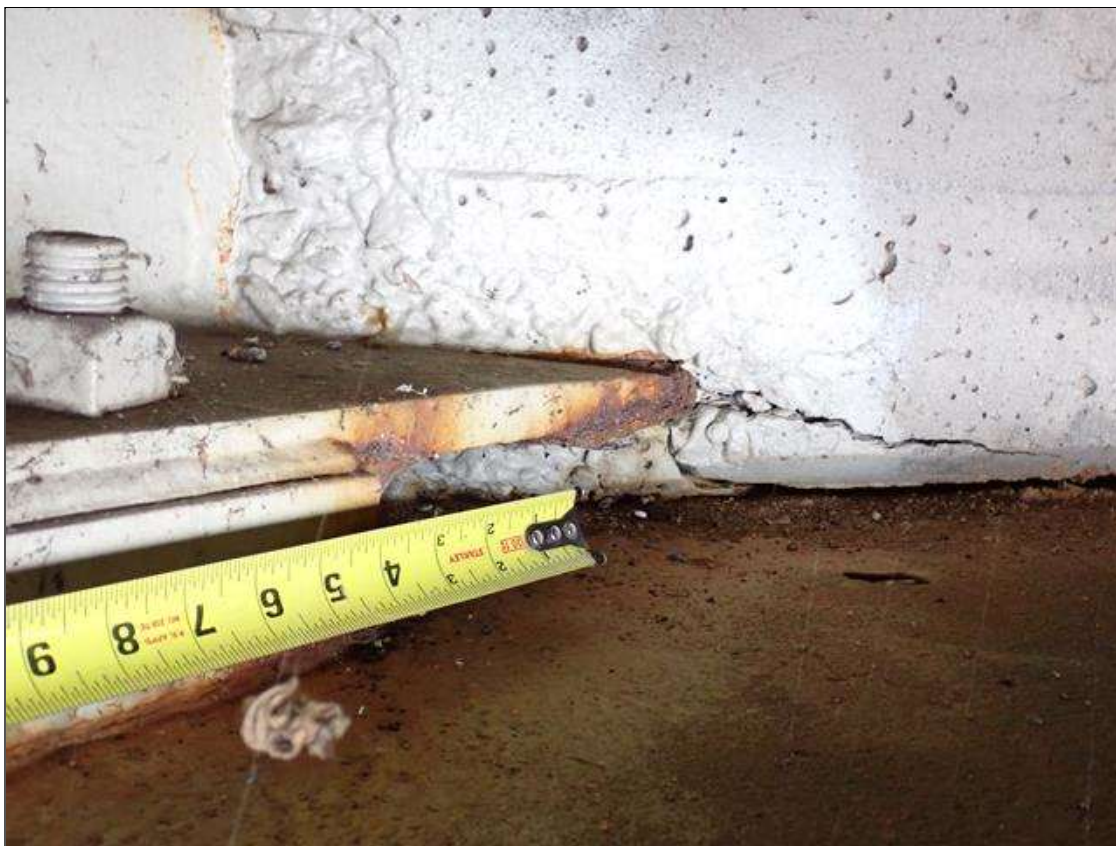
Span 4 Beam 1: at end bent 2, bottom flange, rust scale
