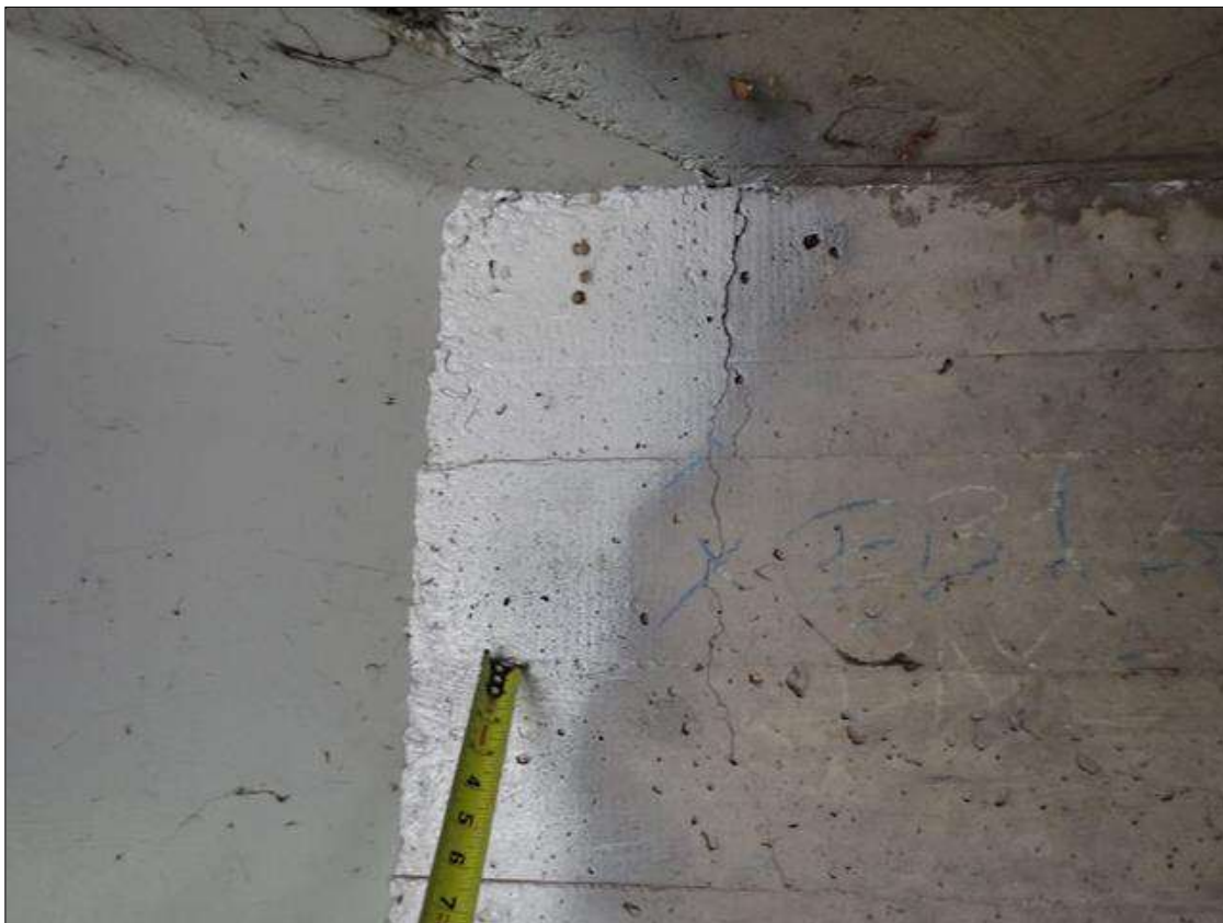
End Bent 2 Abutment: adjacent to beams, spalls/delaminations (up to 18 inch x 10 inch x 1/2 inch deep) with associated cracks (up to 1/16 inch)
