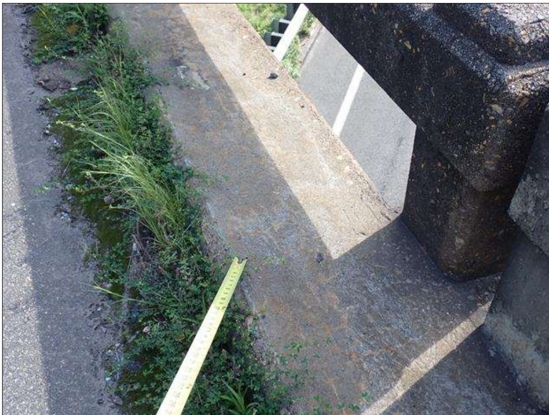
Span 3 Right Bridge Rail: along the safety walk, transverse cracks (up to 1/32 inch) and map cracks (hairline) at random
