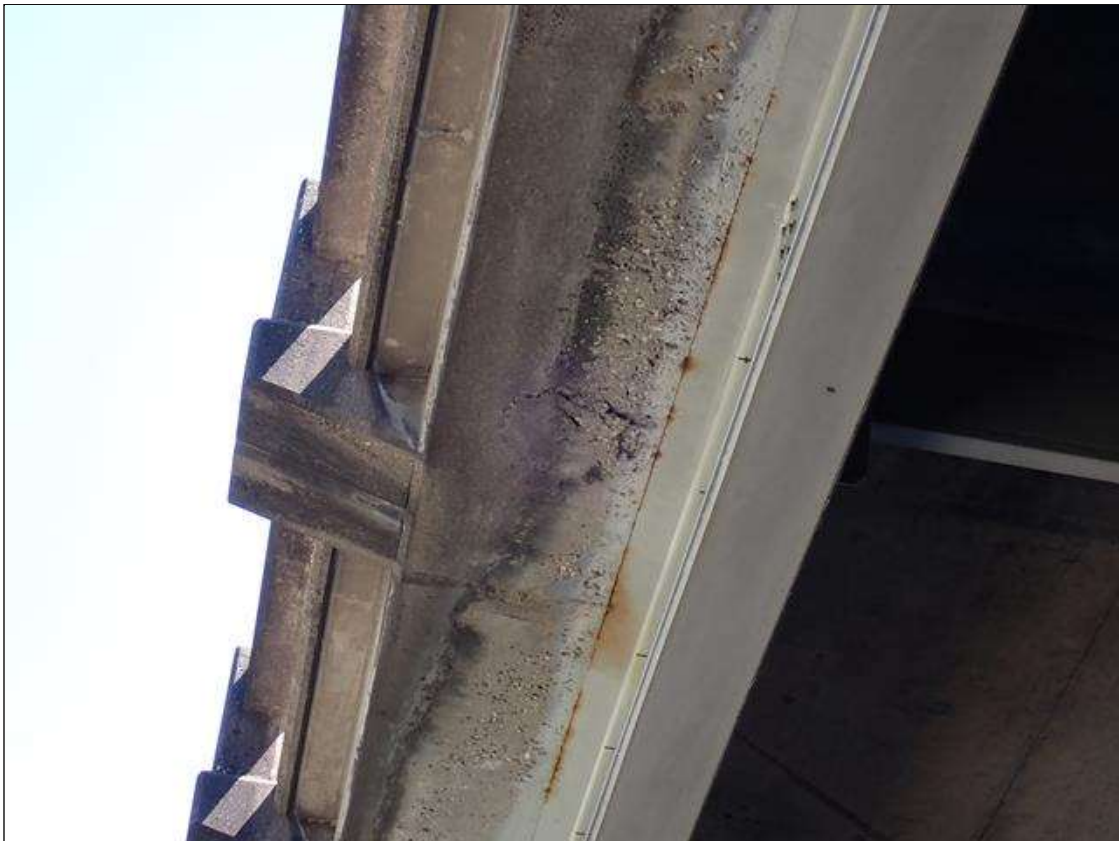
Span 2 Deck: (PAR) both overhangs, delaminations (approximately 1 foot diameter) with cracks (up to 1/8 inch); some areas over travel lanes
