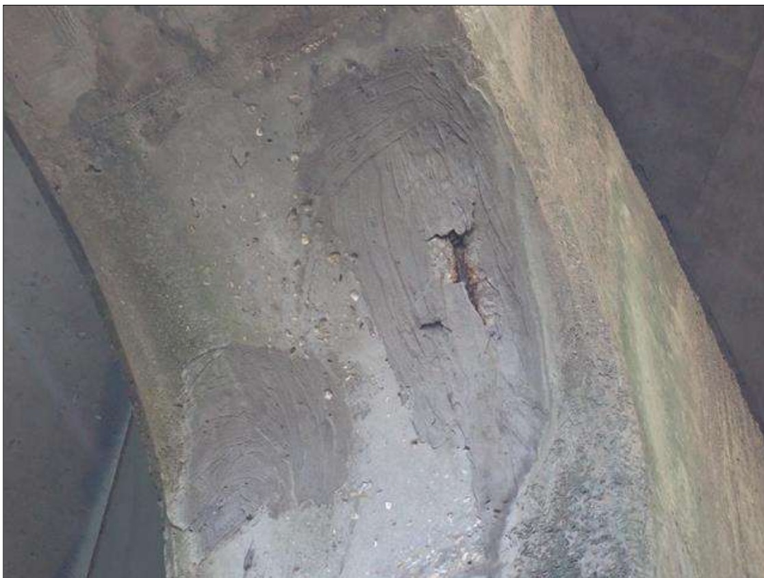
Bent 1 Cap 1: underside, at east end, unsound patched areas (up to 2 feet x 1 foot x 1 inch deep) with exposed rusted rebar
