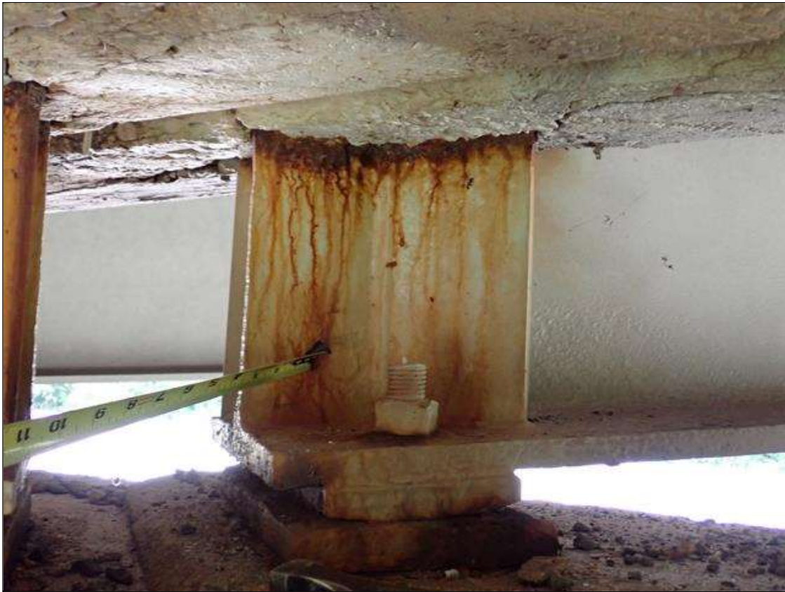
Span 3 Beam 2: at bent 3, painted over section loss: web adjacent to diaphragm and upper web (9/16 inch average remaining x 5 inch x 1 inch); lower web (9/16 average remaining x 5 inch x 3 inch) with adjacent pitting (up to 1/8 inch deep) with corrosion reinitiated
