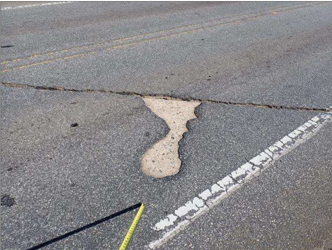
Span 3 Wearing Surface: (PAR) at bent 2, areas of missing asphalt (up to 3 feet x 2 inches) at random; northbound lane, at bent 3, area of missing asphalt (3.5 feet x 2 feet)
