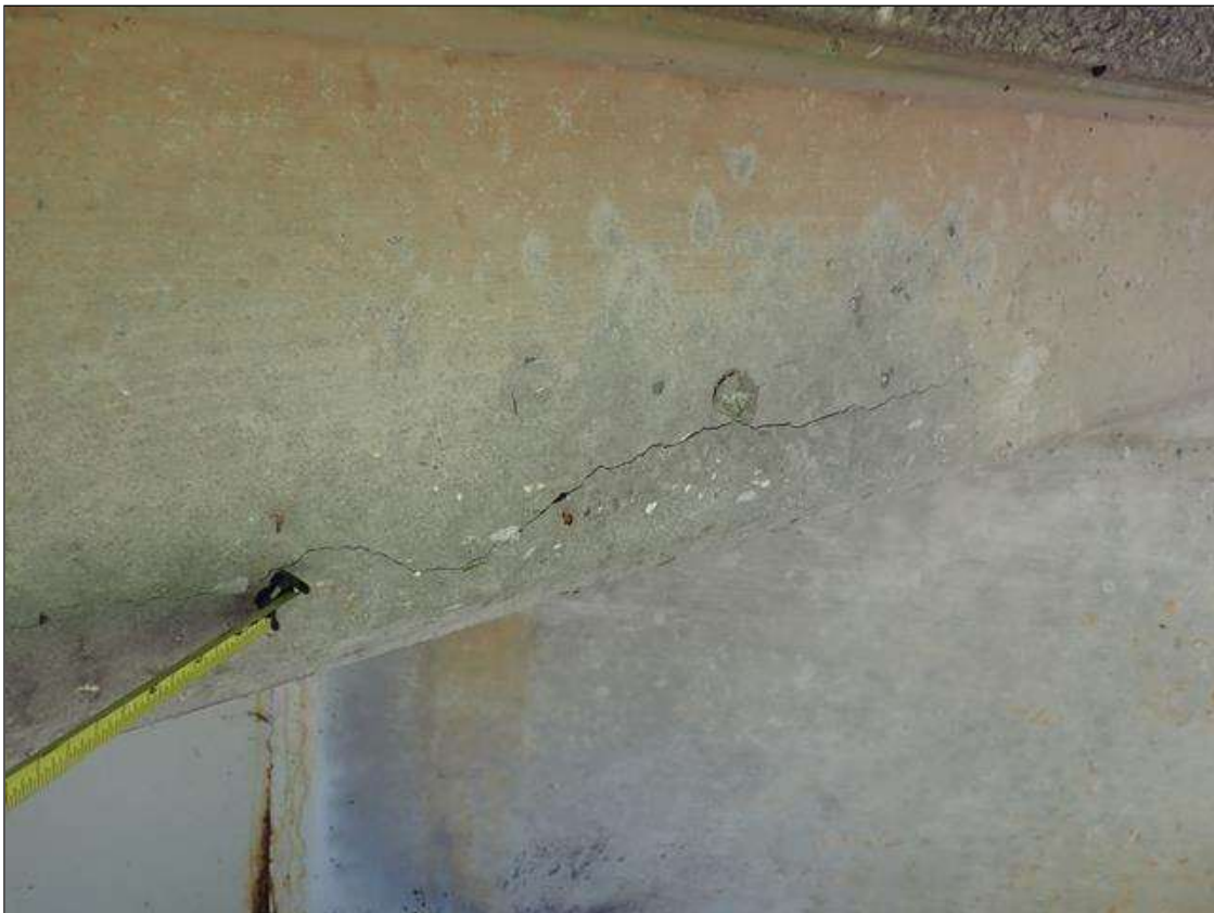
Span 1 Deck: left overhang, near end bent 1, longitudinal crack (1/32 inch x 3 feet)
