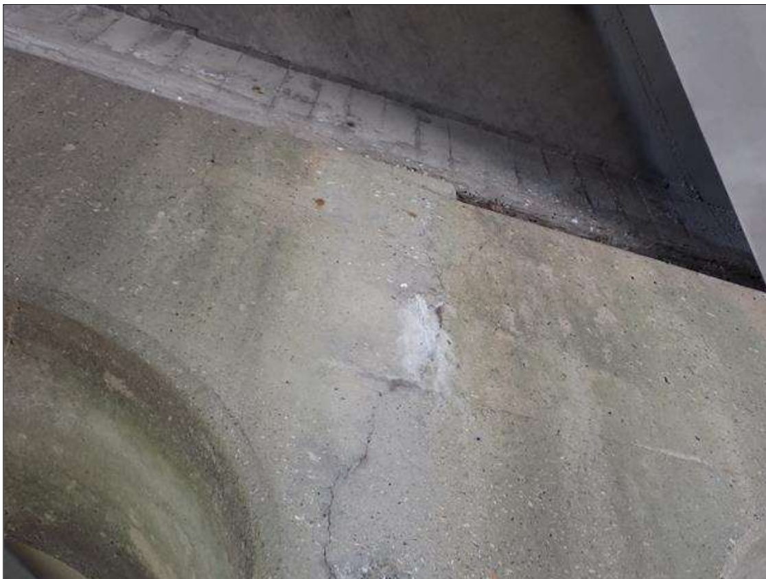
Bent 3 Cap 1: (PAR) UP TO 1/32 INCH MAP CRACKING, SOME WITH EFFLORESCENCE AND RUST STAINS, AT RANDOM THROUGHOUT
