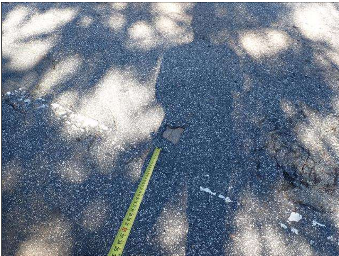
Span 4 Wearing Surface: (PAR) throughout wearing surface, scattered areas of missing asphalt (up to 5 inch diameter)
