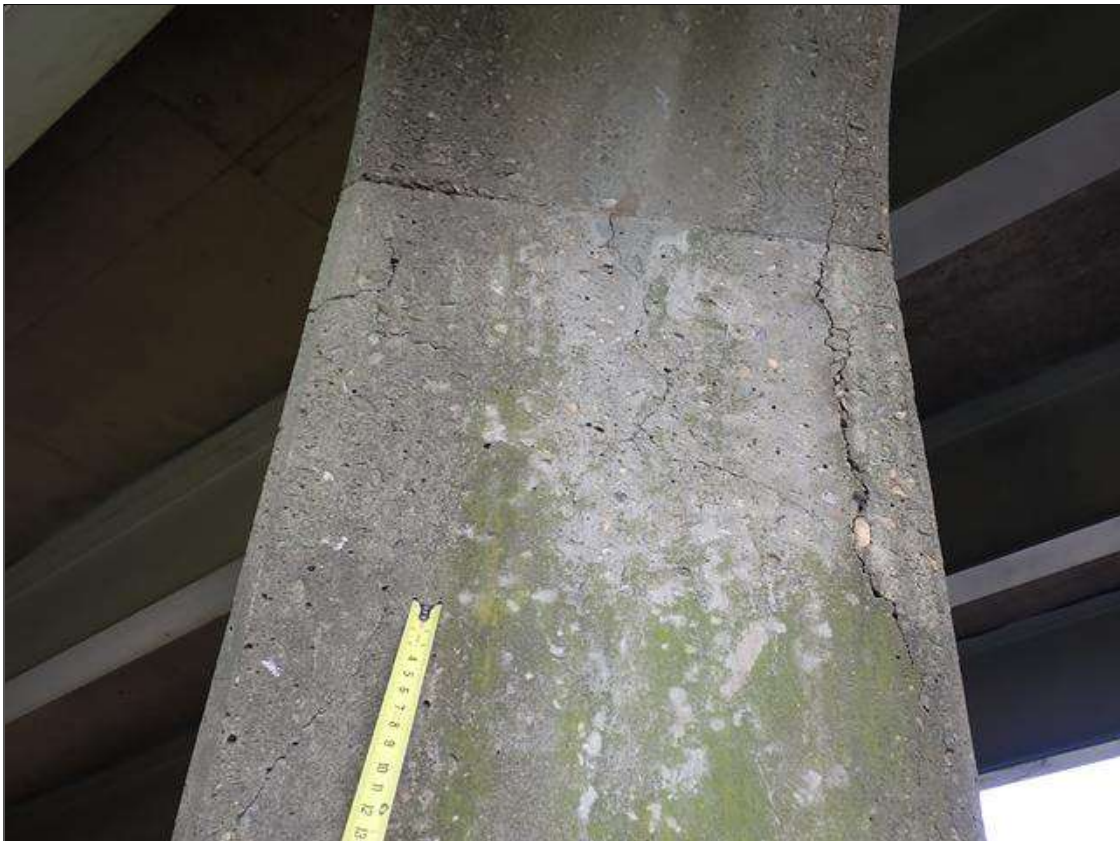
Bent 3 Pile 1: UP TO 1/8 INCH x 6 FOOT VERTICAL CRACKS AND UP TO 1/32 INCH MAP CRACKS AT RANDOM THROUGHOUT, some with efflorescence, some with adjacent delamination, up to 4 foot x 1 foot
