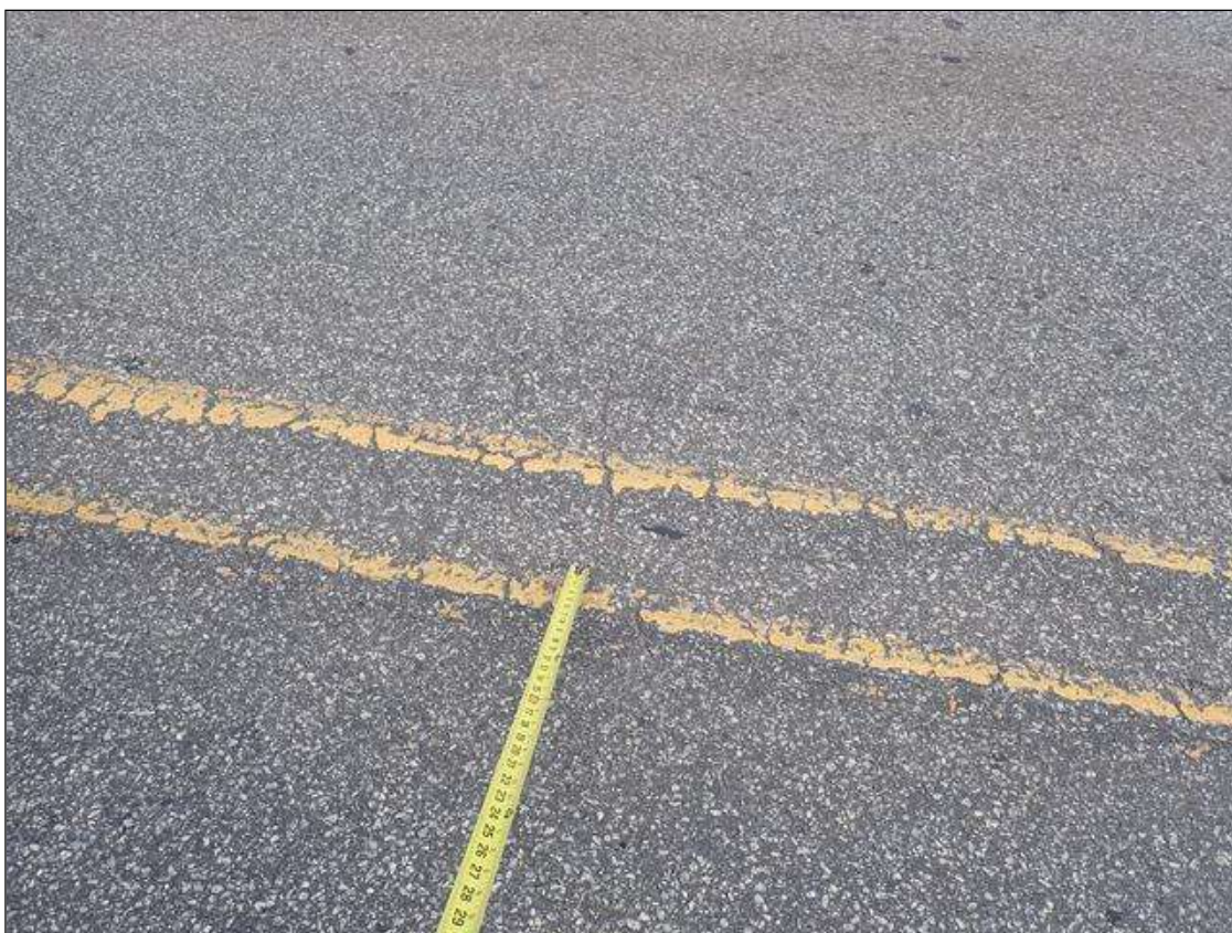
Span 1 Wearing Surface: SPAN 1 WEARING SURFACE HAS SCATTERED TRANSVERSE AND LONGITUDINAL CRACKS UP TO 1/8 INCH.
