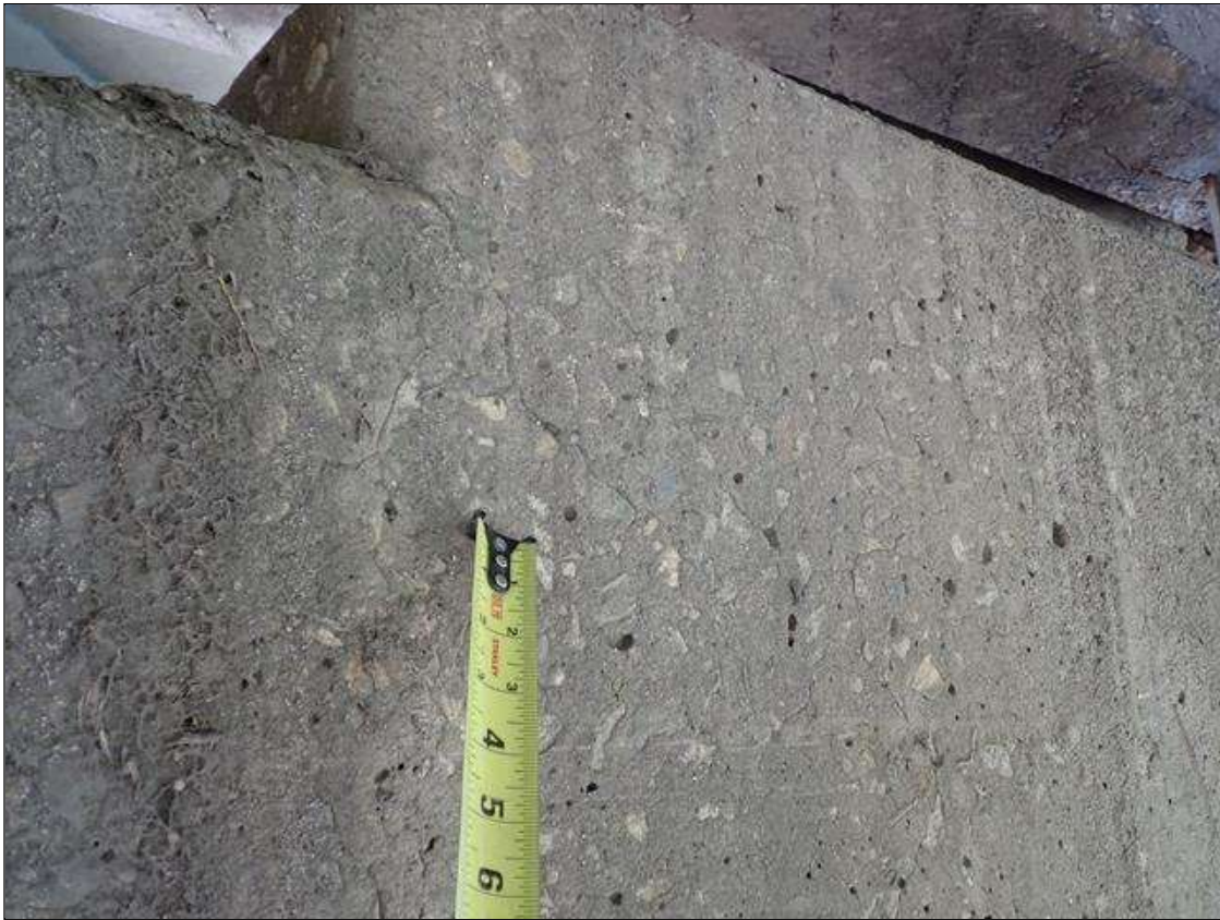
Bent 2 Cap 1: south and north face, areas of map cracks (hairline) at random
