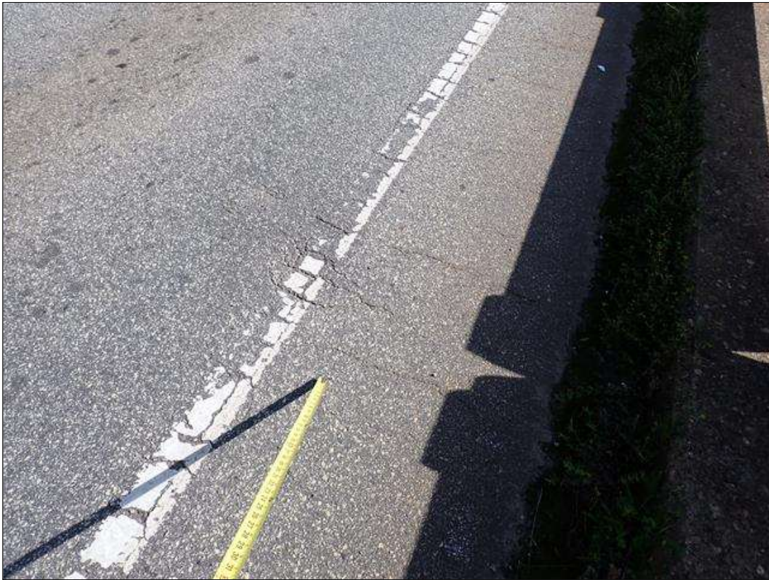
Span 3 Wearing Surface: SPAN 3 WEARING SURFACE HAS SCATTERED MAP/TRANSVERSE AND LONGITUDINAL CRACKS UP TO 1/8 INCH.
