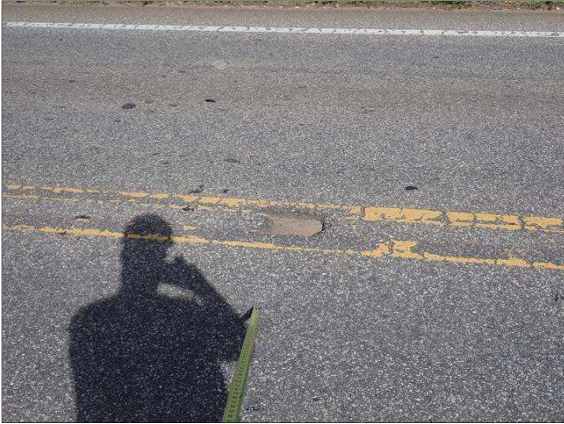
Span 2 Wearing Surface: (PAR) along centerline of roadway, approximately 25 feet from bent 2, spall (11 inch x 6 inch x full depth)
