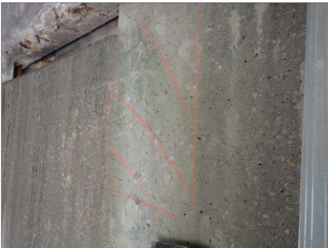
Bent 2 Cap 1: North face over column 2, vertical crack, 1/32 inch x full height, extends up from vertical crack on column 2, with adjacent delamination, 26 inch x 15 inch
