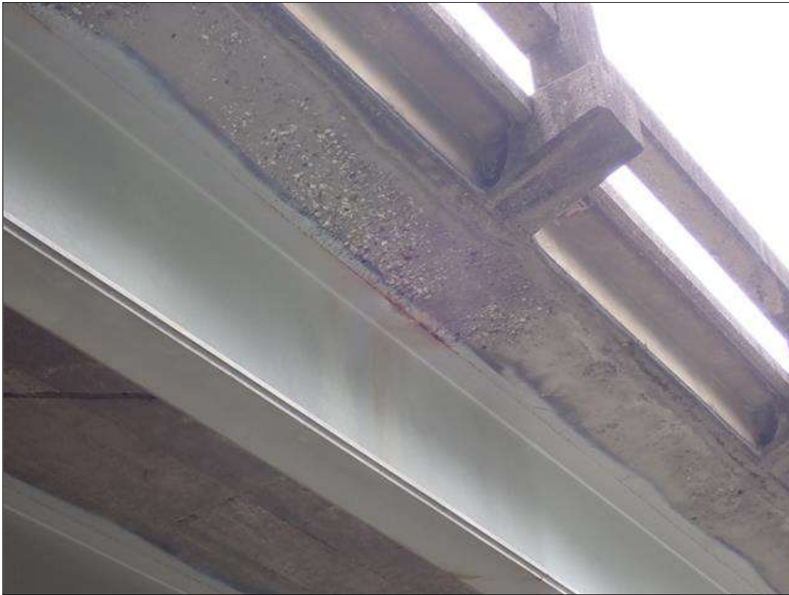
Span 3 Beam 1: along the edge of the top flange, surface rust at random
