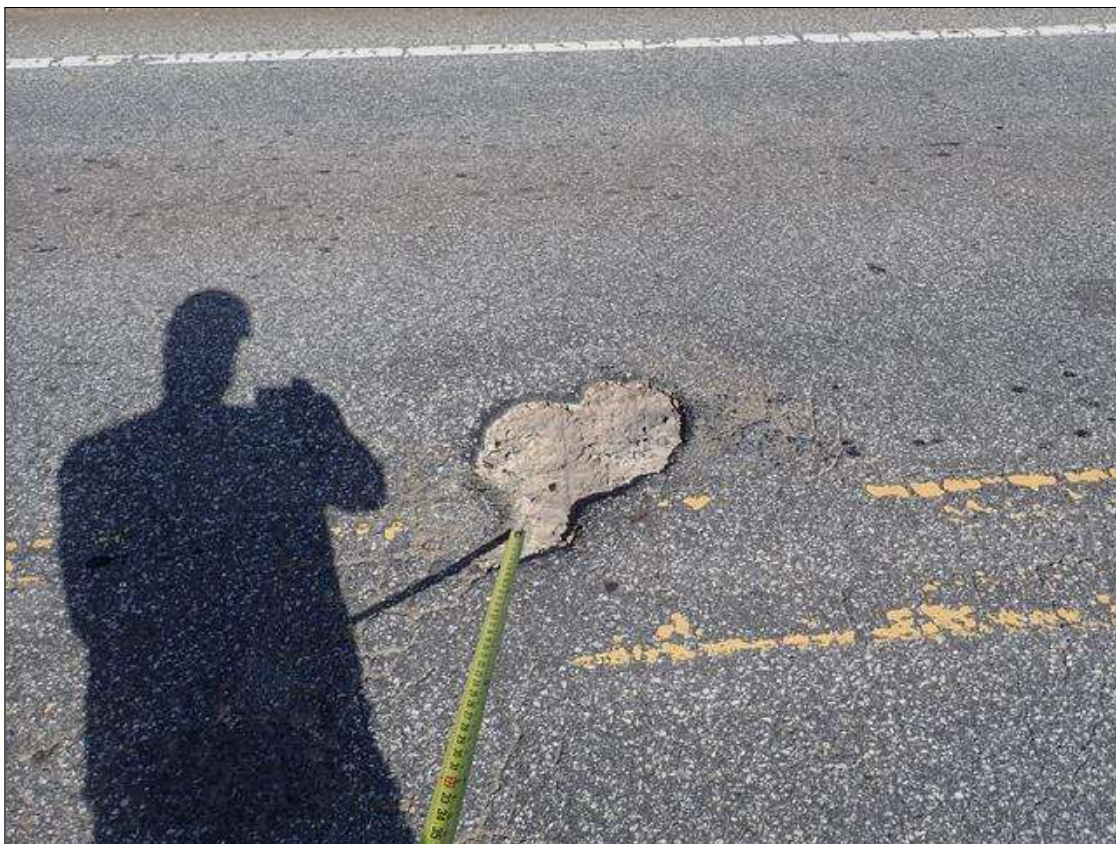
Span 3 Deck: (PAR) top of deck near bent 2, spall (2 feet x 15 inch x 1.5 inch deep) with exposed rusted rebar at area of missing asphalt
