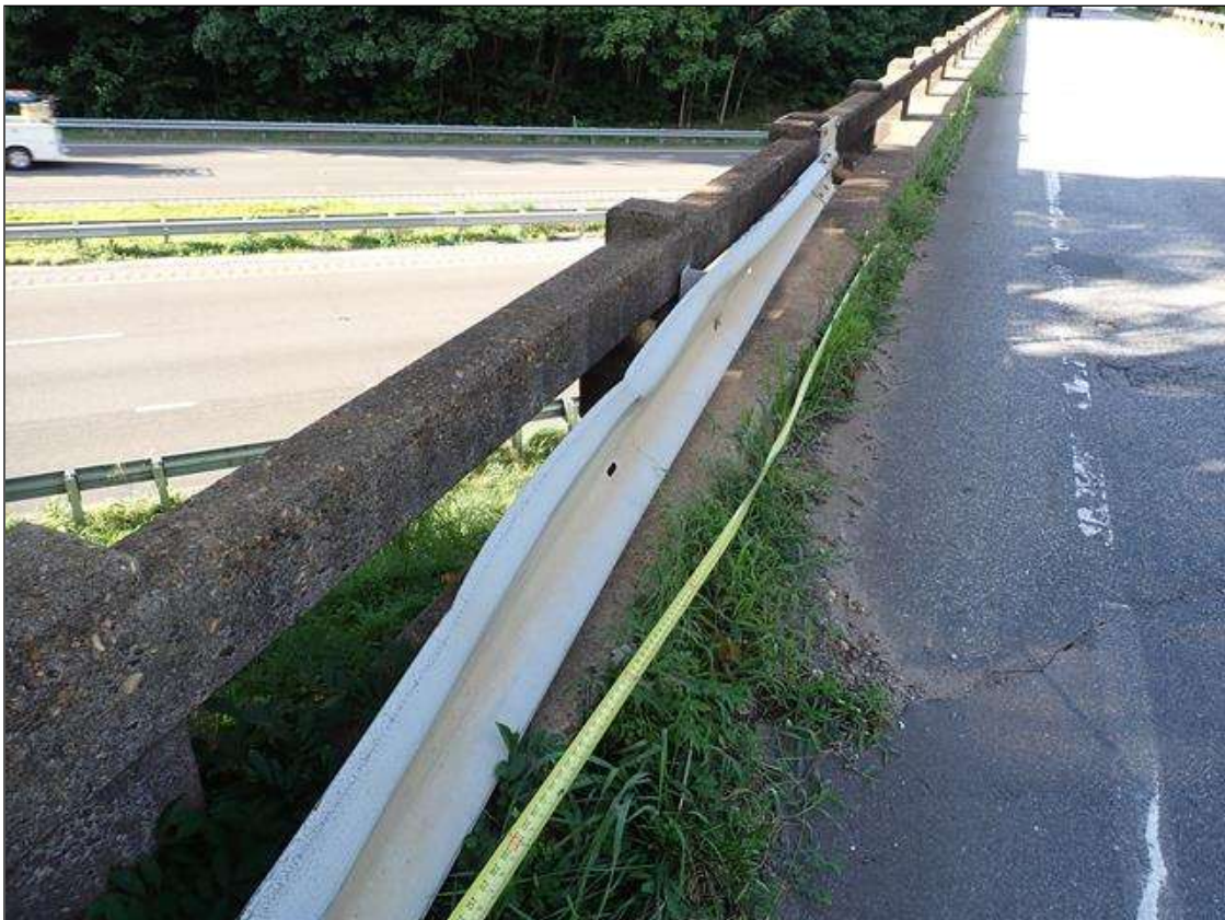
(PAR) northeast guardrail and transition, areas of impact damage (up to 15 feet long, 30 feet total)
