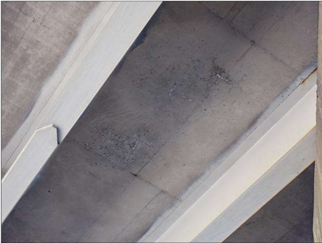
Span 2 Deck: underside of deck, in all bays and overhangs, areas of map cracks (hairline), some with efflorescence; both overhangs, transverse cracks (up to 1/32 inch x full width) at random
