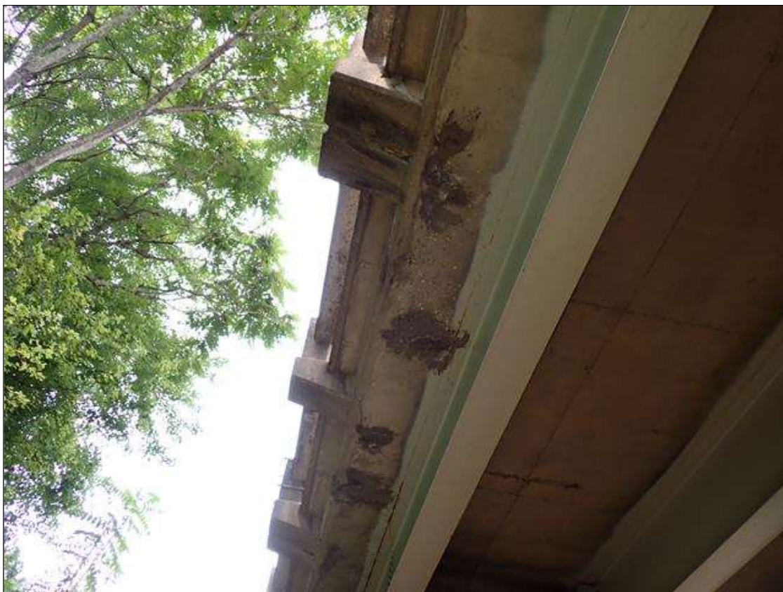
Span 4 Deck: MULTIPLE SOUND PATCHES UP TO 2.5 FEET x 2 FEET IN UNDERSIDE OF WEST OVERHANG AT RANDOM THROUGHOUT.
