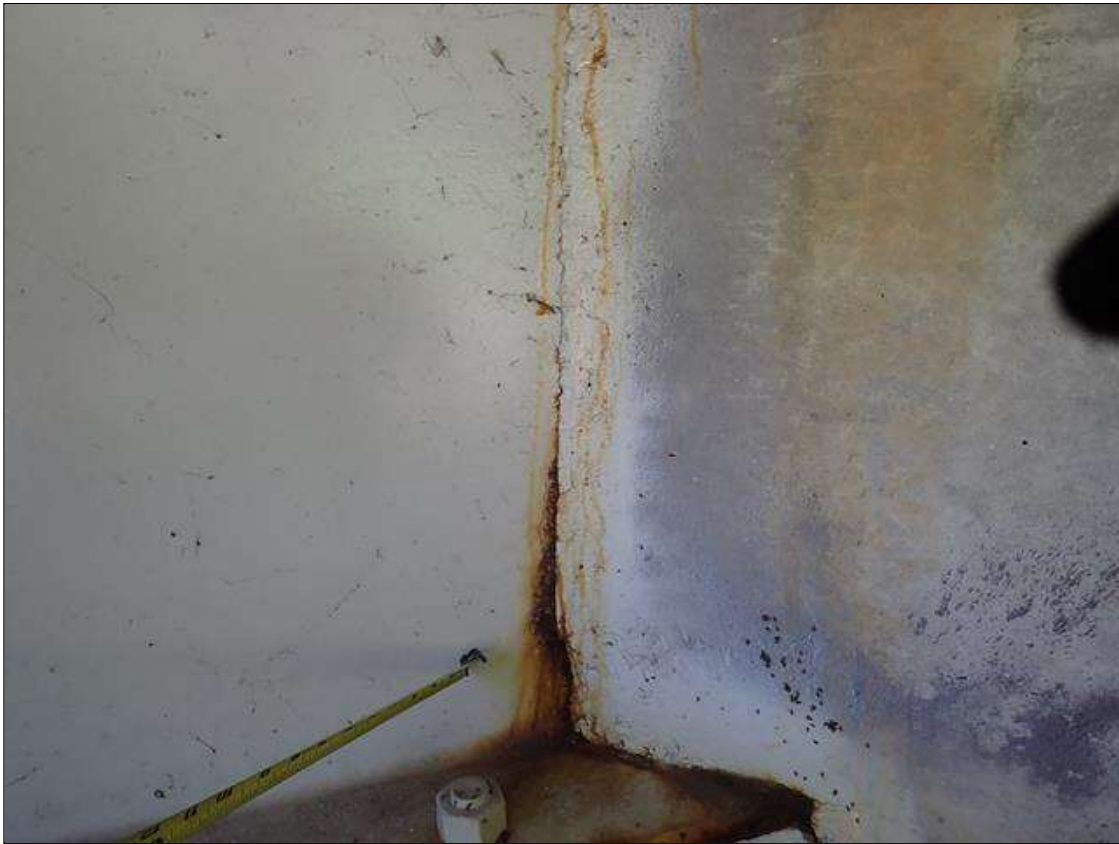
Span 1 Beam 1: at end bent 1, web and bottom flange, rust scale
