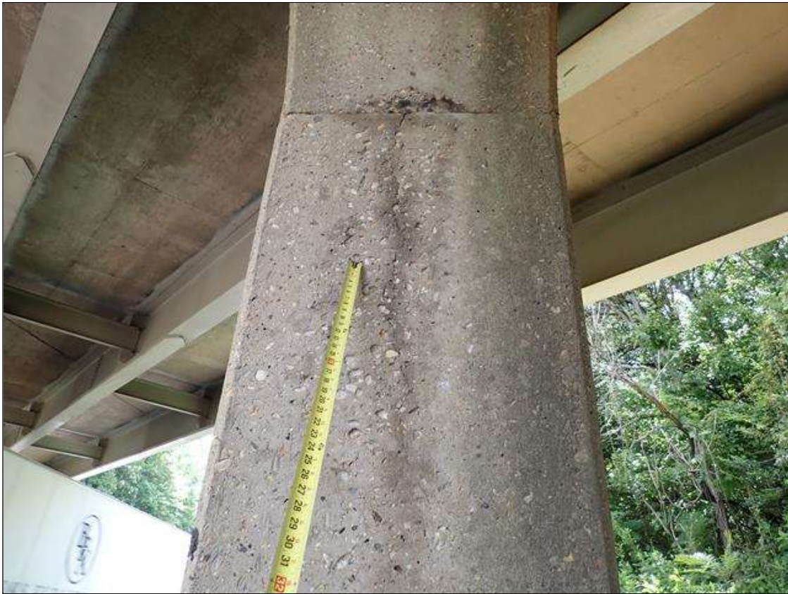
Bent 3 Pile 2: south, north and east faces, multiple vertical cracks, up to 4 feet x 1/16 inch wide with adjacent delaminations (4 feet x 10 inch)
