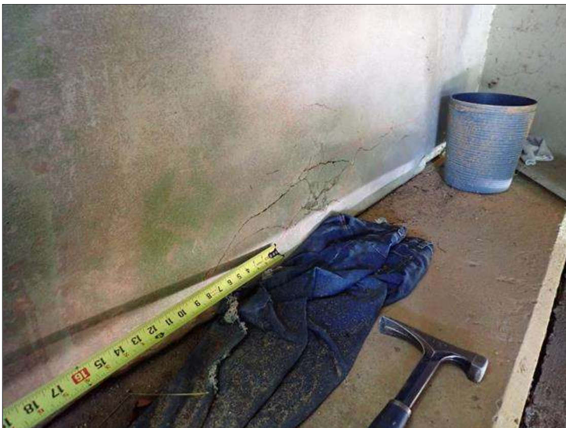
End Bent 1 Abutment: right side of beam 4, delamination 3.5 feet x up to 1 foot, with cracks up to 1/16 inch
