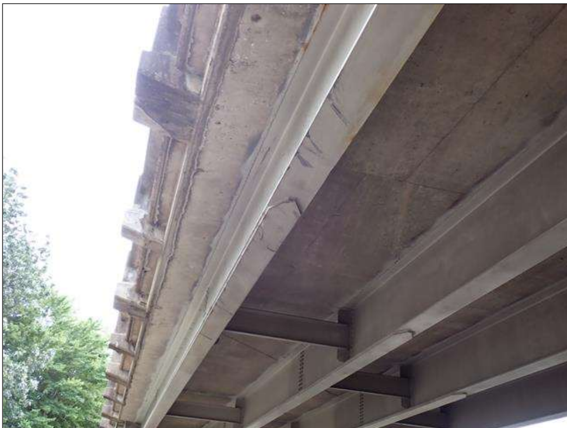
Span 3 Beam 4: over I-40 westbound, right travel lane, bottom flange and cover plate, impact scrapes/gouges (up to 1/4 inch deep)
