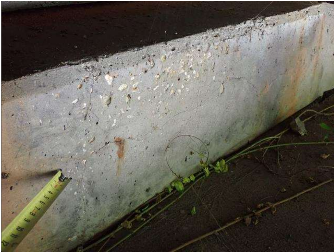
End Bent 2 Cap 1: (PAR) along the length of the cap, vertical and longitudinal cracks (up to 1/32 inch x 5 feet), some with rust stains at random
