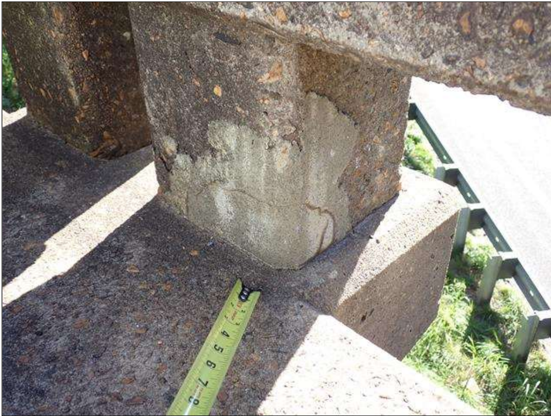
Span 4 Right Bridge Rail: rail post 3, patched area (8 inch x 10 inch) with hairline cracks
