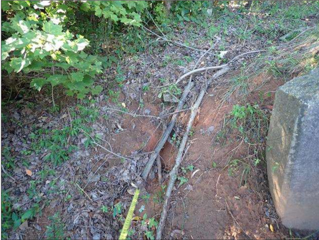
(PAR) east side of span 1, extending from behind southeast wingwall to toe of end bent 1 slope protection, erosion channel (approximately 100 feet long x 3 feet long x 1.5 feet deep) undermining slope protection (up to 1 foot high x 1.5 foot deep)
