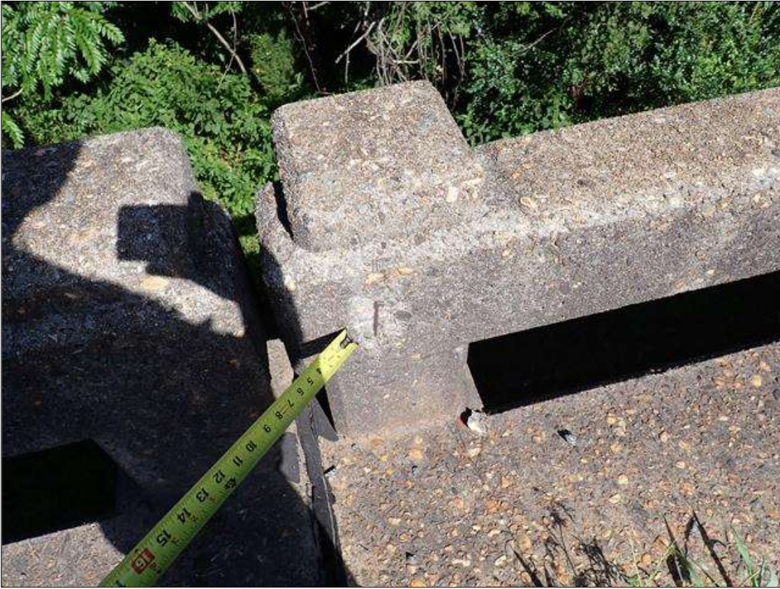
Span 4 Left Bridge Rail: at rail post 1, spall (5 inch x 3 inch x 1/2 inch deep) with exposed rusted rebar
