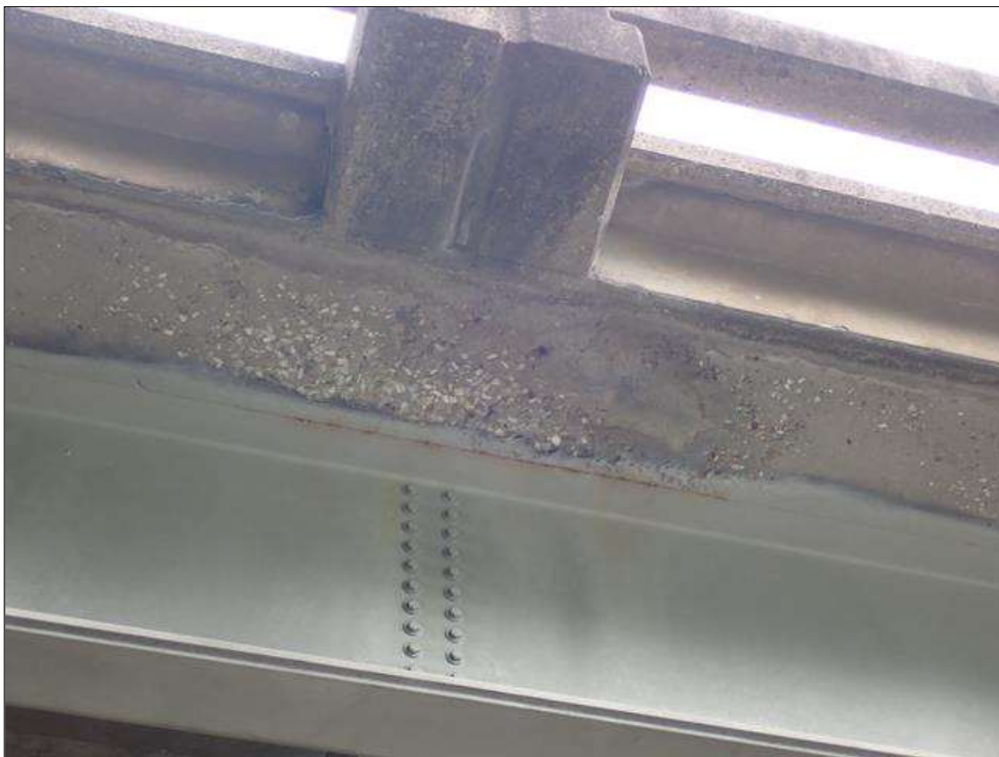
Span 3 Deck: left overhang, areas of poor consolidation (up to 1/2 inch deep) at random
