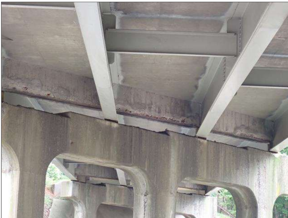
Span 3 Deck: at bents 2 and 3, end diaphragms in all bays, unsound patches/delaminations/spalls (up to full bay width x 8 inch x 1.5 inch deep), some with exposed rusted rebar
