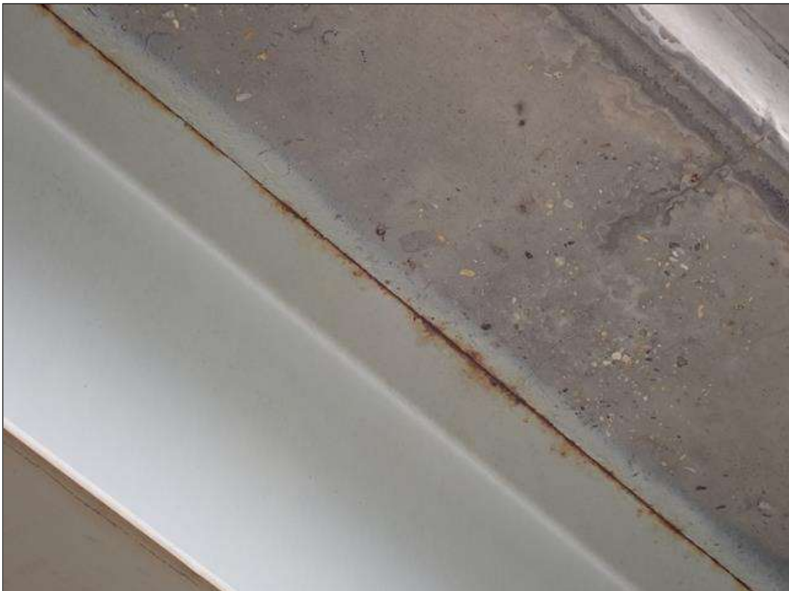
Span 4 Beam 4: along the edge of the top flange, surface rust at random
