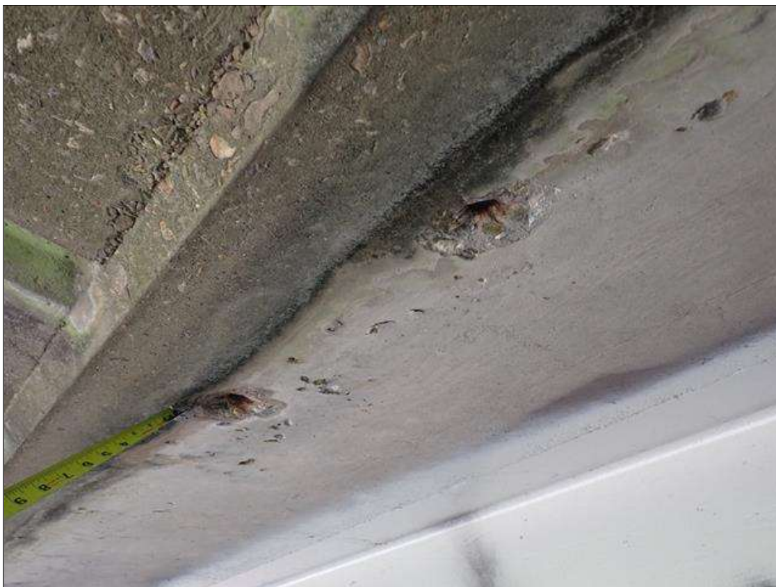
Span 1 Deck: (PAR) left and right overhangs, near end bent 1, spalls (up to 6 inch x 4 inch x 1 inch deep) with exposed rusted rebar
