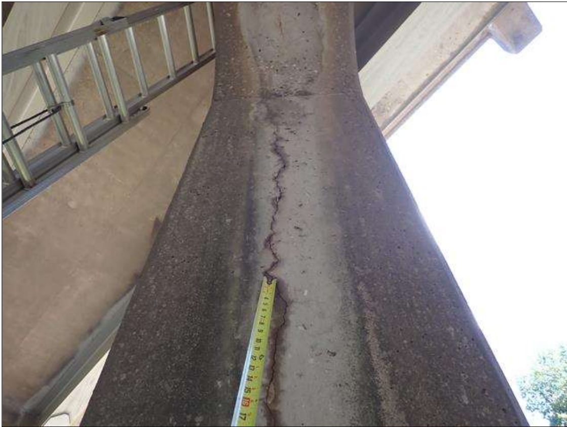
Bent 2 Pile 3: (PAR) UP TO 1/8 INCH VERTICAL CRACKS WITH RUST STAINS AT RANDOM THROUGHOUT with adjacent delaminations up to 6 feet x 1 foot
