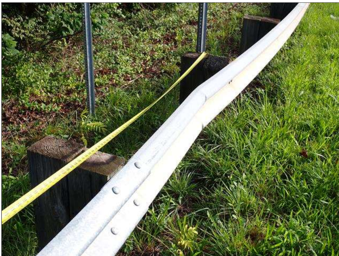
(PAR) southwest guardrail, areas of impact damage (up to 15 feet long, 30 feet total)
