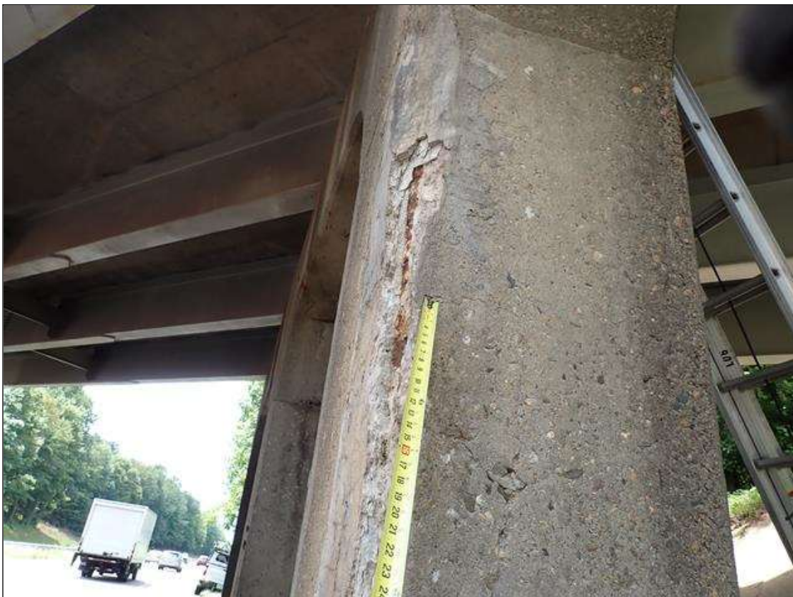
Bent 3 Pile 3: (PAR) at Southeast corner, failed patch/delamination/spall, 8 feet x up to 2 feet x 2.5 inches deep, with exposed rusted primary reinforcing
