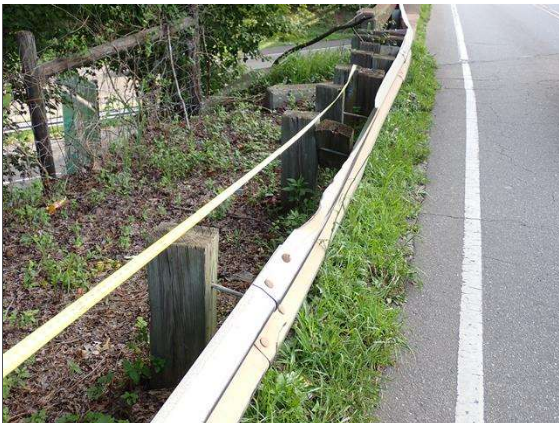
(PAR) southwest guardrail, areas of impact damage (up to 15 feet long, 30 feet total)
