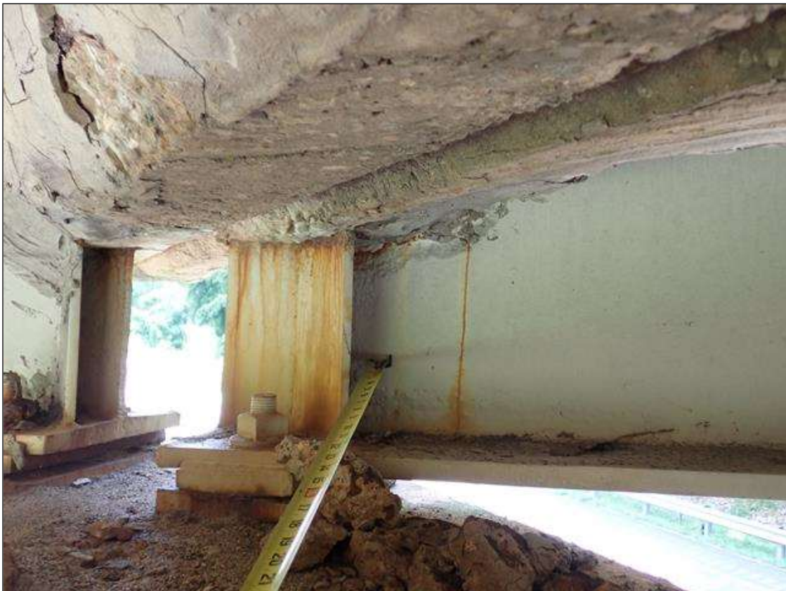
Span 2 Beam 4: at bent 2, painted over section loss: web adjacent to diaphragm (9/16 inch average remaining x 9 inch x 2 inch); lower web (9/16 inch average remaining x 1.5 feet x 3 inches) with corrosion reinitiated
