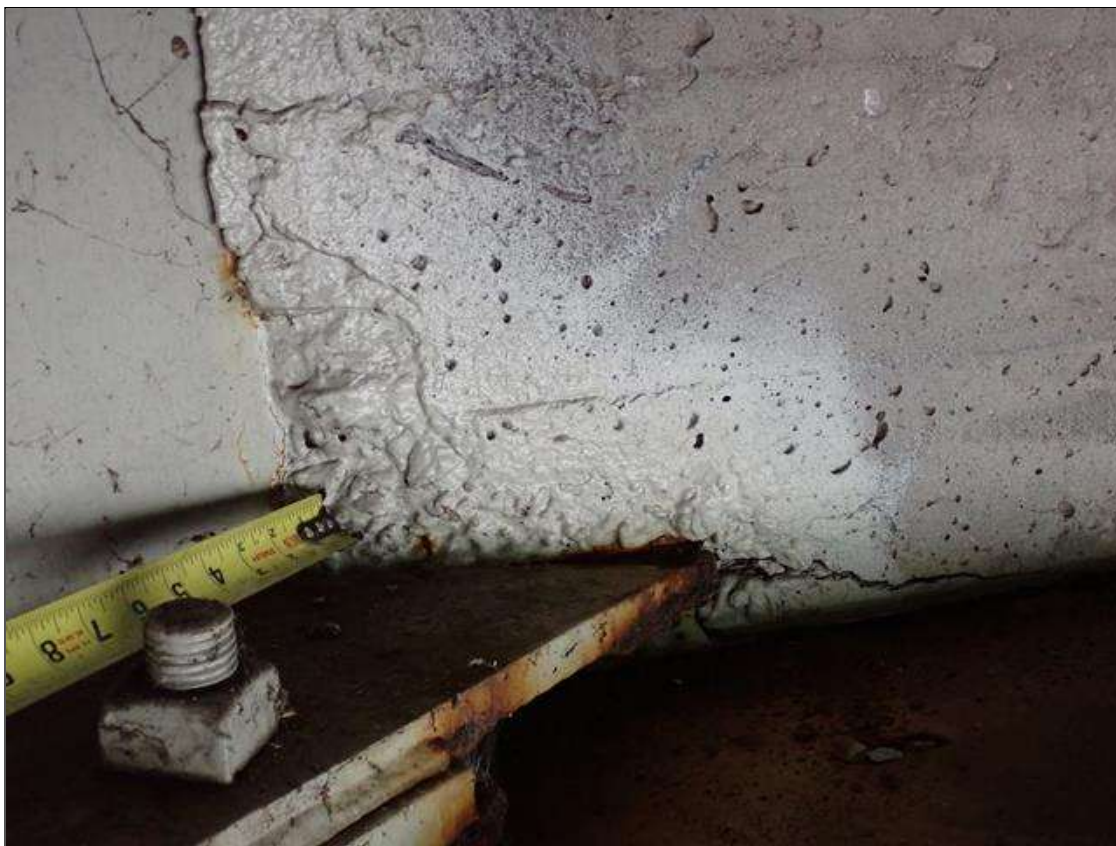
End Bent 2 Abutment: adjacent to beams, spalls/delaminations (up to 18 inch x 10 inch x 1/2 inch deep) with associated cracks (up to 1/16 inch)
