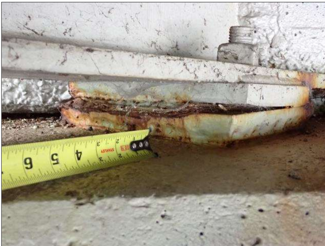
Span 4 Beam 1 - Far Bearing 1: painted over section loss (up to 1/4 inch deep) with corrosion reinitiated
