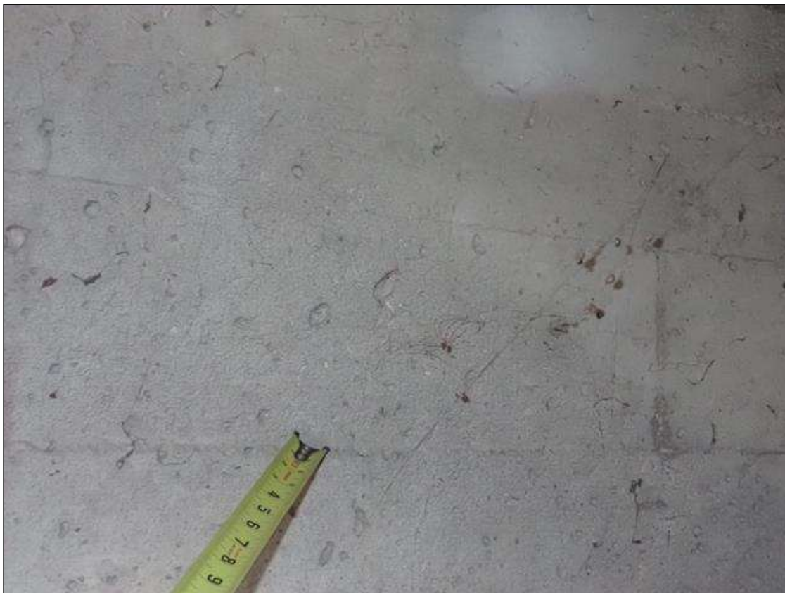
End Bent 2 Abutment: along the abutment, areas of map cracks (hairline) at random
