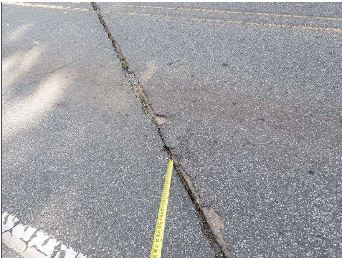
Span 1 Wearing Surface: 2023 previously repaired, previously noted as: 1 FOOT X 4 FOOT AREA OF MISSING ASPHALT WEARING SURFACE IN SOUTHBOUND LANE AT BENT 1
