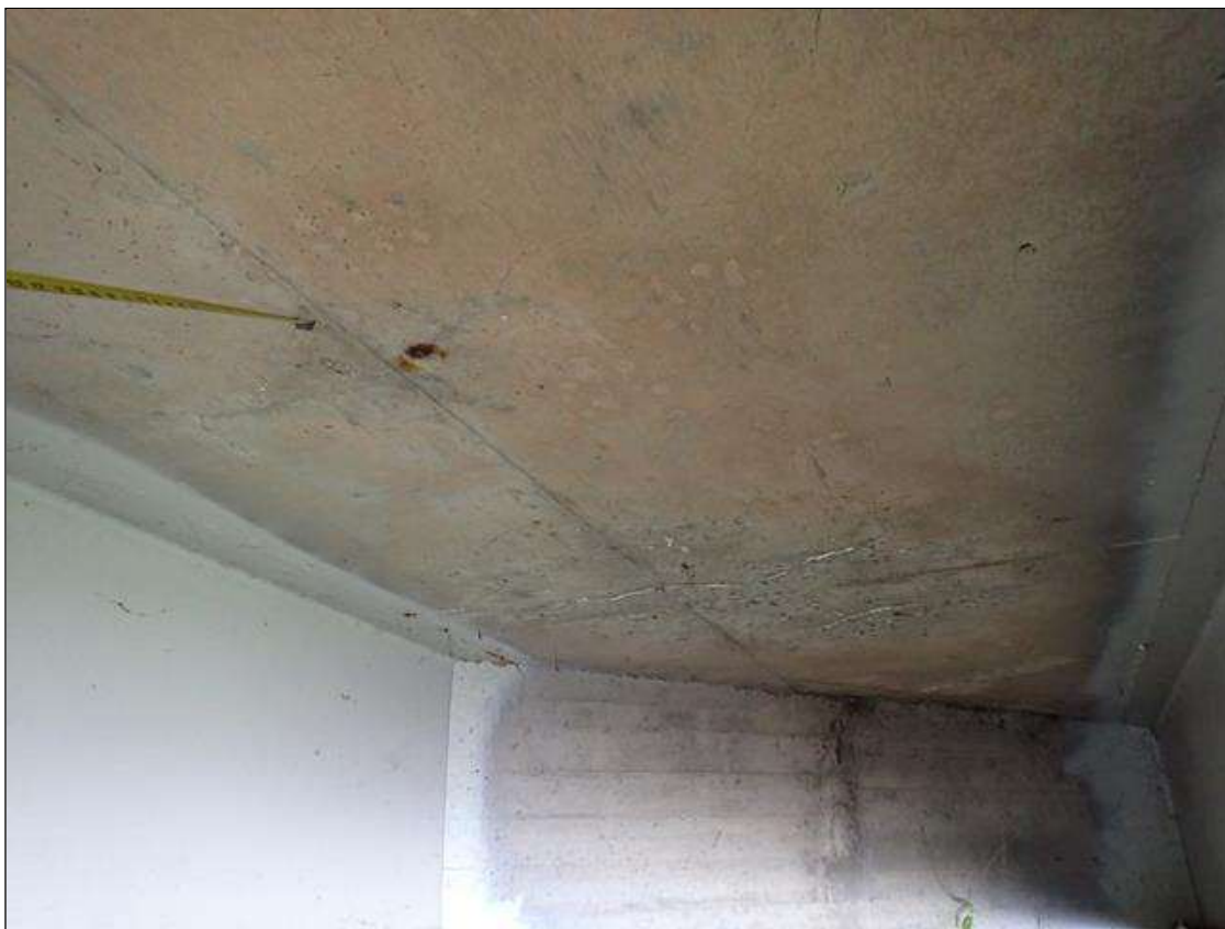
Span 4 Deck: (PAR) throughout underside of deck, transverse cracks (up to 1/32 inch x full bay width) and map cracks (hairline), some with efflorescence buildup and rust stains at random
