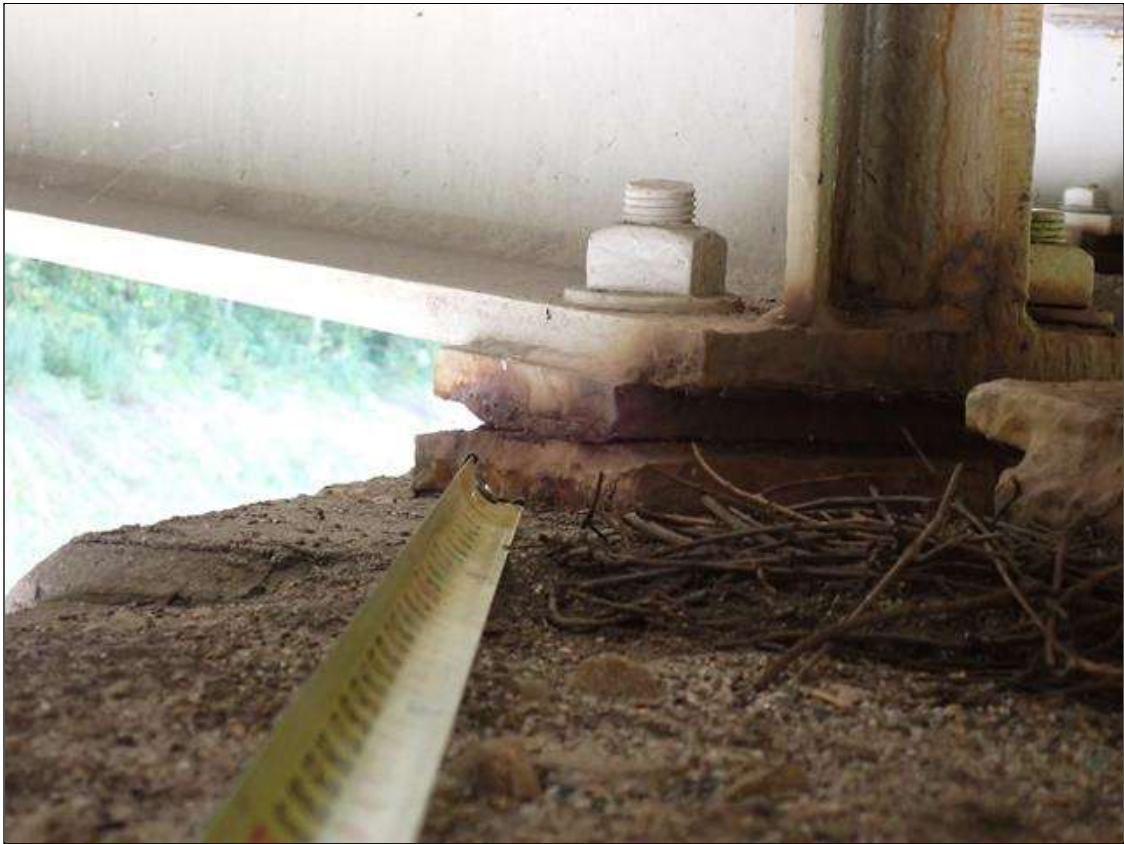
Span 2 Beam 3 - Far Bearing 3: painted over section loss (up to 3/16 inch deep) with corrosion reinitiated; pack rust
