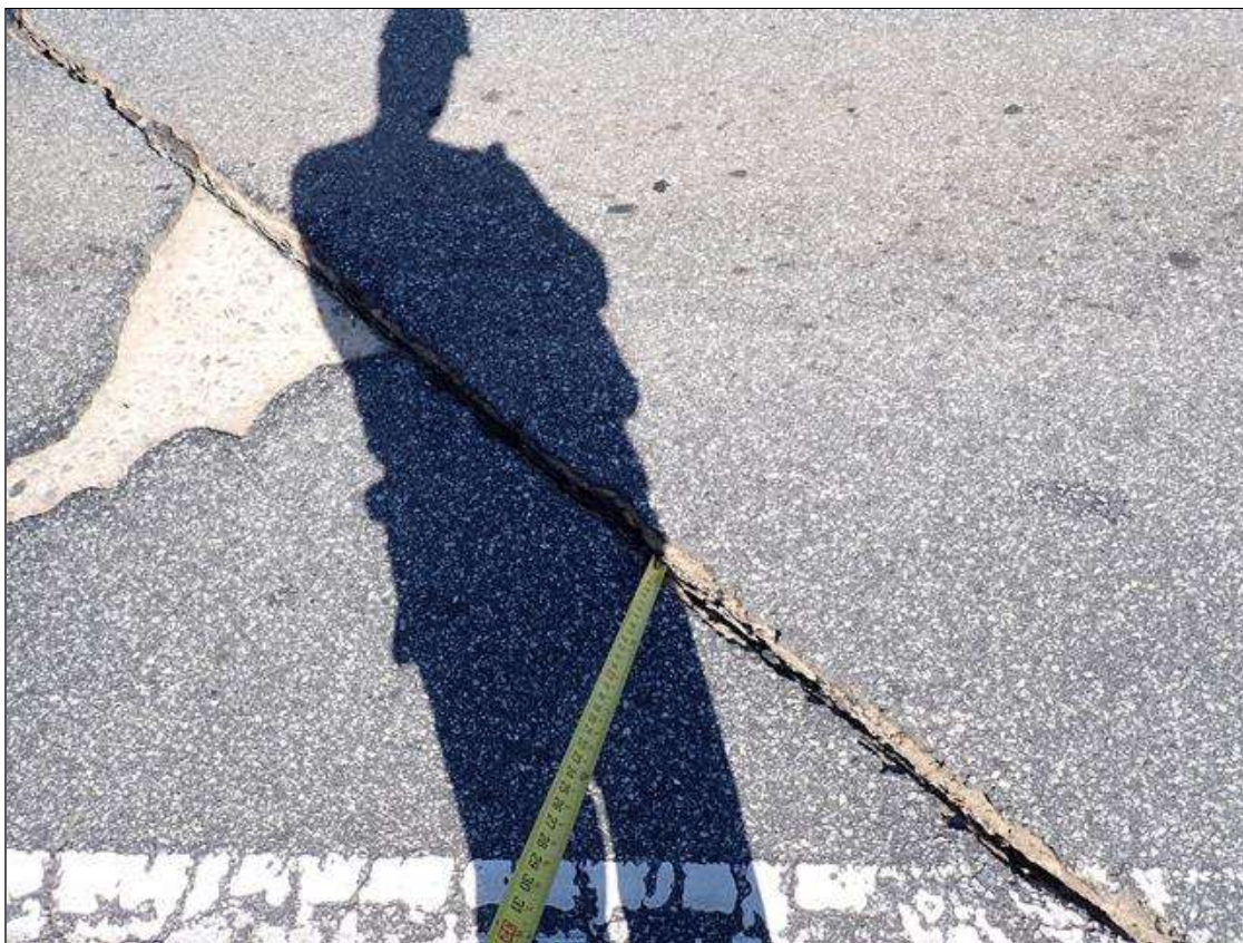
Span 4 Wearing Surface: (PAR) at bent 3, areas of missing asphalt (up to 2 feet x 2 inch) at random
