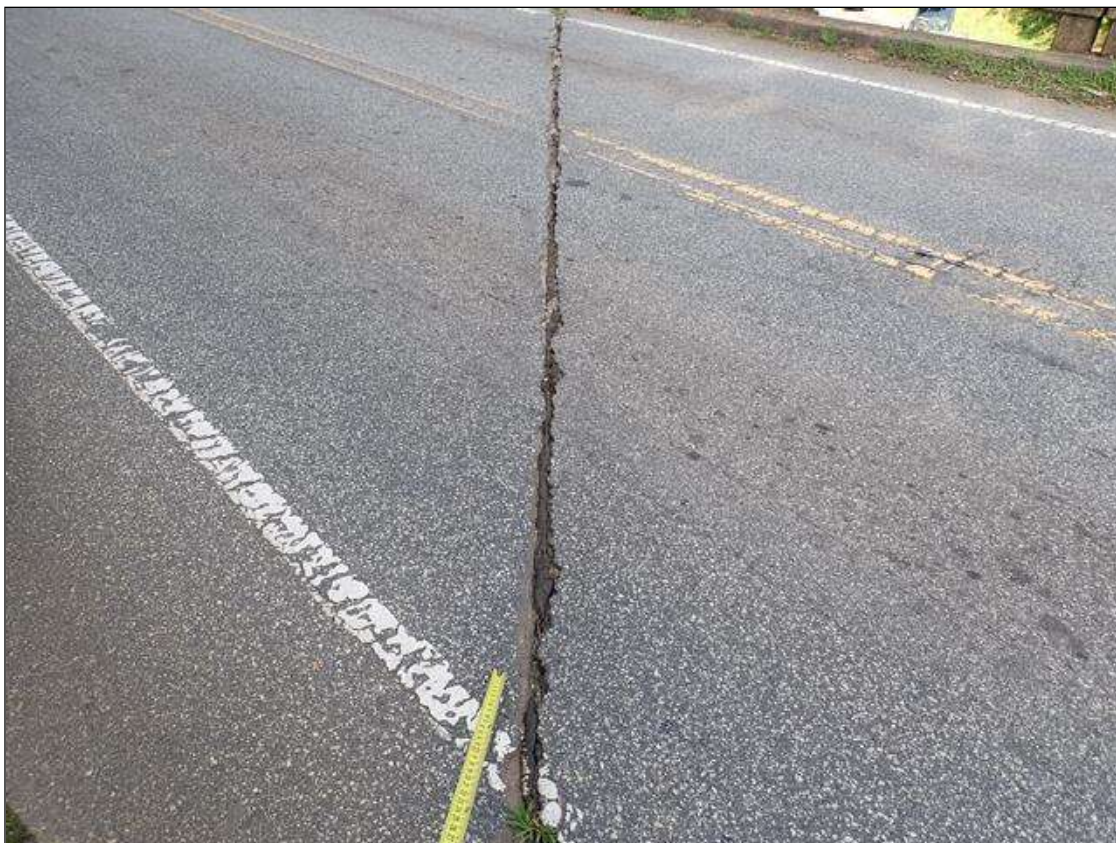
Span 2 Bent 1 Joint: along the length of the joint, seal deteriorated (full length)
