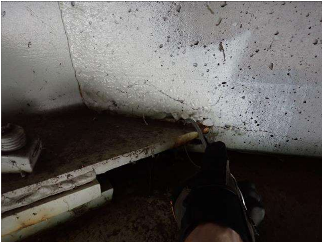
Span 4 Beam 2: at end bent 2, bottom flange, behind bearing, painted over section loss (0.83 inch average remaining x 2 inches) with corrosion reinitiated
