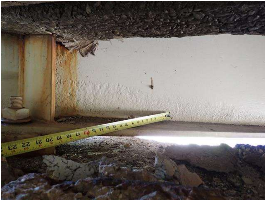
Span 2 Beam 1: at bent 1, lower web, painted over section loss (9/16 inch average remaining x 5.5 feet x up to 10 inches) with corrosion reinitiated
