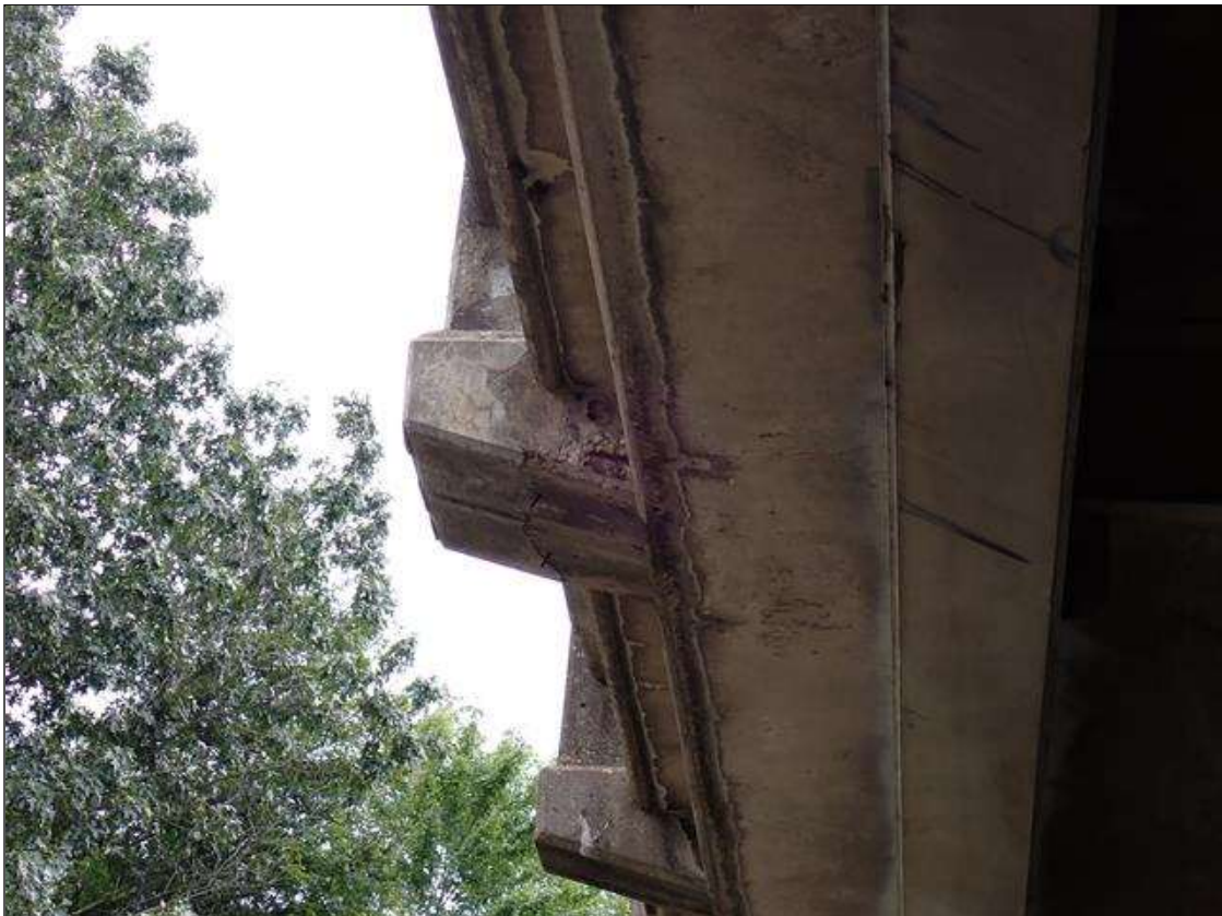
Span 3 Right Bridge Rail: underside of rail section and outriggers, shallow rebar at random
