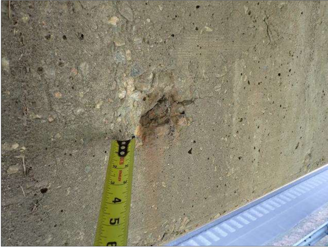
Bent 2 Cap 1: north face, below bay 3, spall (4 inch diameter x 1 inch deep) with exposed rusted rebar
