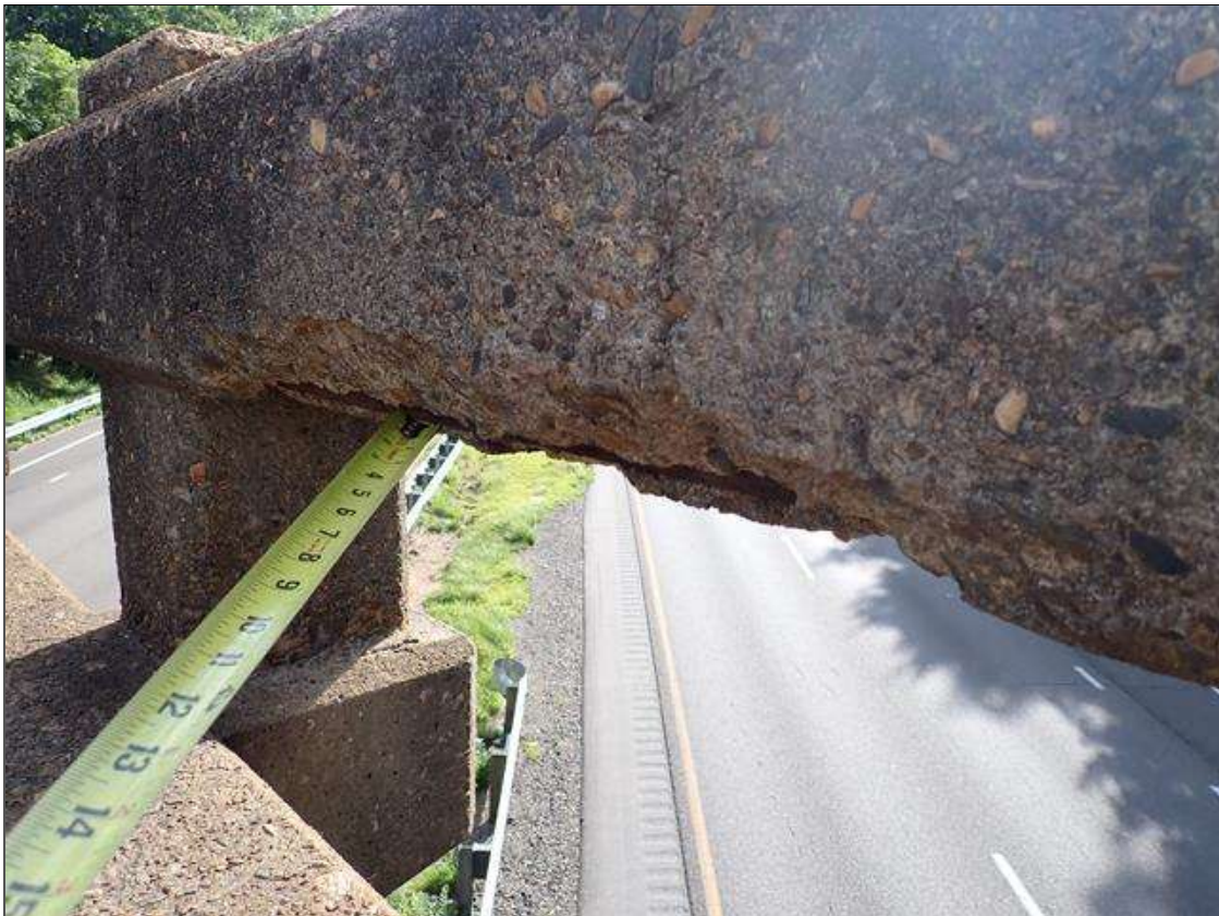
Span 2 Right Bridge Rail: rail section 2 from bent 2, spall (27 inch x 4 inch x 1.5 inch deep) with exposed rusted rebar; adjacent post with diagonal crack (up to 1/32 inch x 6 inches)
