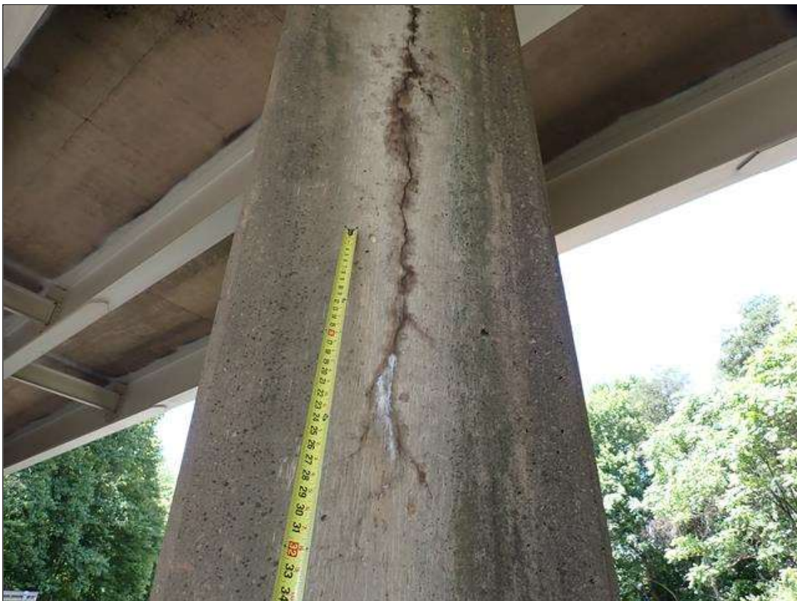
Bent 2 Pile 2: 6 FOOT X UP TO 1/16 INCH VERTICAL CRACK WITH EFFLORESCENCE EAST FACE AT BOTTOM OF CAP. (SIMILAR ON WEST FACE)
