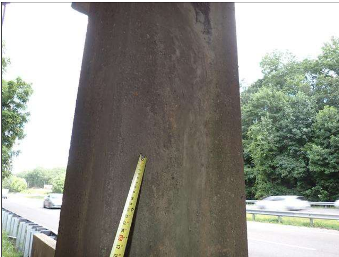
Bent 3 Pile 3: WEST FACE AND SOUTHWEST AND NORTHWEST CORNERS HAVE PATCHED AREAS UP TO 8.5 FEET X 1 FOOT WITH SCATTERED MAP CRACKING UP TO 1/32 INCH.
