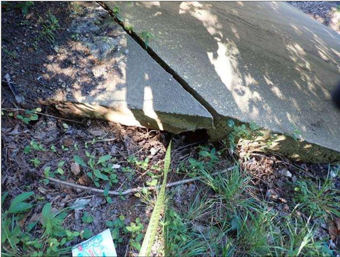
(PAR) east side of span 1, extending from behind southeast wingwall to toe of end bent 1 slope protection, erosion channel (approximately 100 feet long x 3 feet long x 1.5 feet deep) undermining slope protection (up to 1 foot high x 1.5 foot deep)
