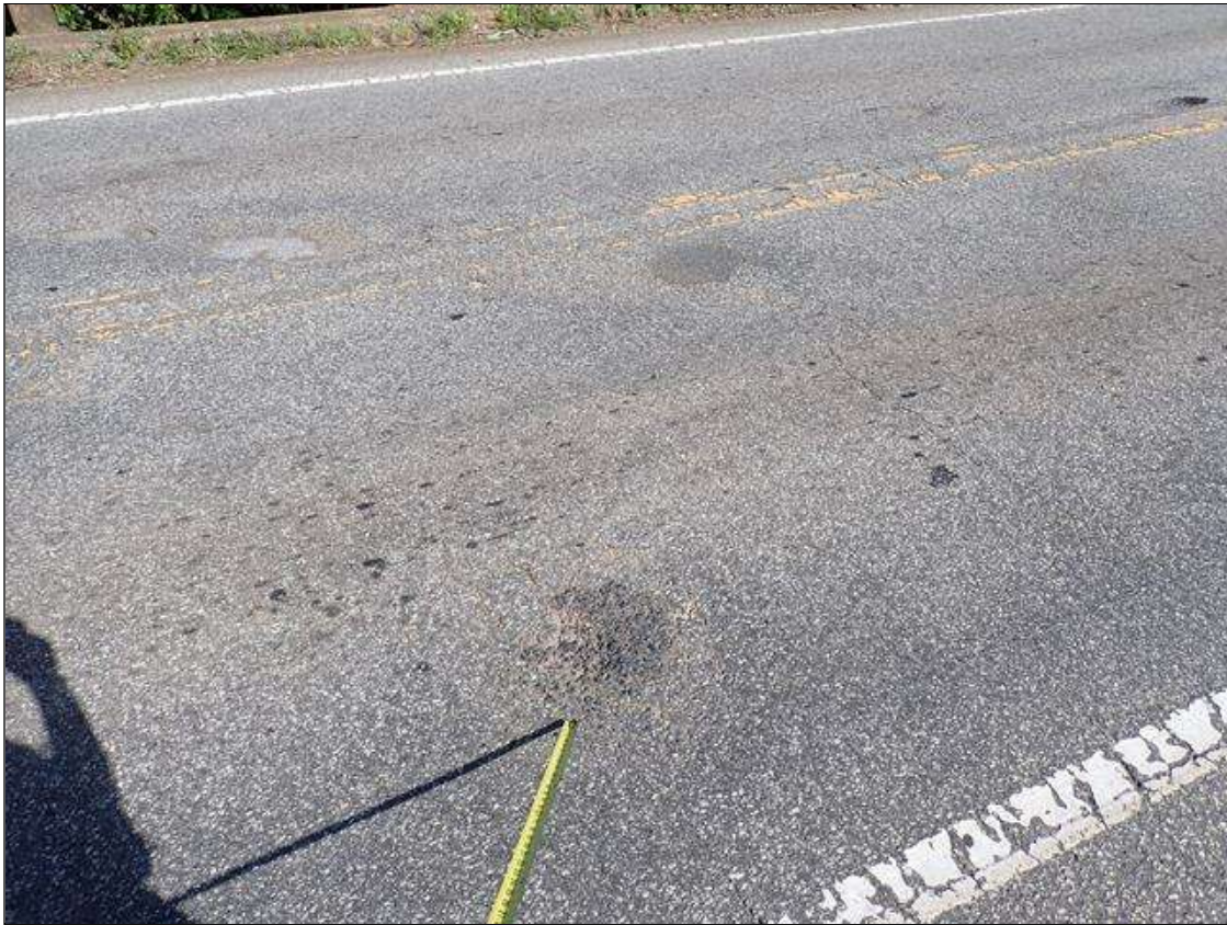
Span 3 Wearing Surface: WEARING SURFACE HAS SCATTERED PATCHED AREAS WITH SOME MAP CRACKING.
