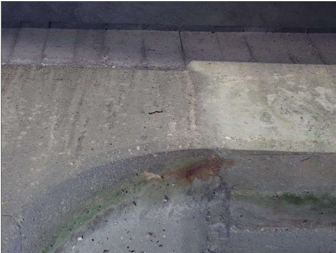
Bent 1 Cap 1: (PAR) BENT 1 CAP HAS SCATTERED CRACKS UP TO 1/32 INCH, SOME WITH RUST STAINS.
