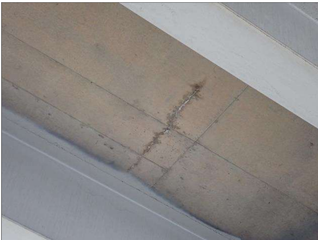
Span 4 Deck: (PAR) throughout underside of deck, transverse cracks (up to 1/32 inch x full bay width) and map cracks (hairline), some with efflorescence buildup and rust stains at random
