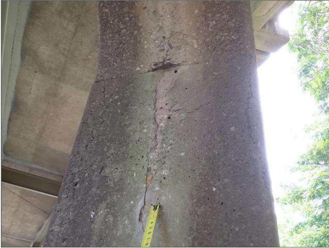
Bent 3 Pile 1: UP TO 1/8 INCH x 6 FOOT VERTICAL CRACKS AND UP TO 1/32 INCH MAP CRACKS AT RANDOM THROUGHOUT, some with efflorescence, some with adjacent delamination, up to 4 foot x 1 foot
