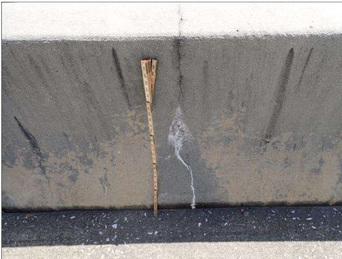
Span 2 Right Bridge Rail: along length of rail, map cracks [hairline] and multiple vertical cracks [up to full height x 1/32 inch], some wrap around, some with efflorescence
