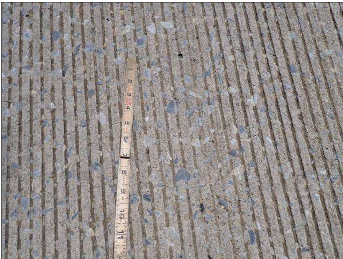
Span 2 Deck: throughout topside of deck, map cracks (hairline) and transverse/longitudinal cracks (up to 1/32 inch x 12 foot) at random
