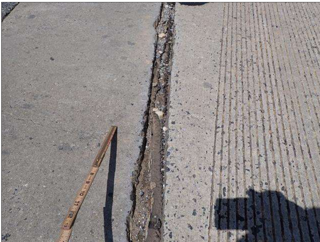
Span 1 Expansion Joint at End Bent 1: along the length of the joint, seal deteriorated/torn and adhesion loss (up to full length x full depth)
