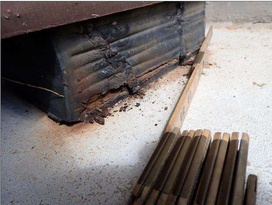
Span 1 Far Bearing 6: (PAR) east face, bulging (up to 1/8 inch high) with tear (10 inch x 1/4 inch wide) exposing steel plate; steel plate, rust scale; southeast corner, loss of bearing (1 inch x 1.5 inch)
