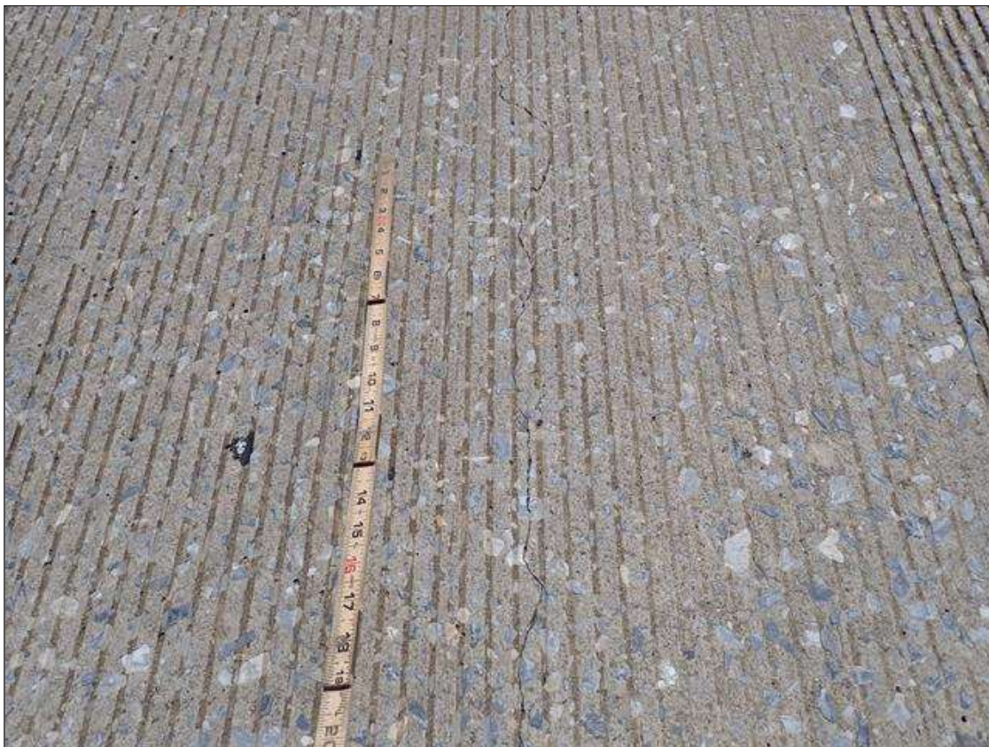
Span 2 Deck: throughout topside of deck, map cracks (hairline) and transverse/longitudinal cracks (up to 1/32 inch x 12 foot) at random
