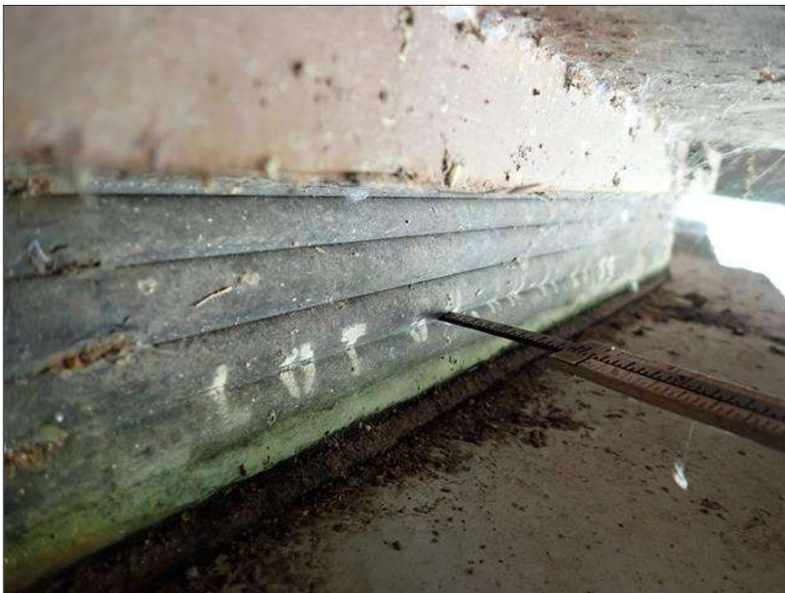
Span 1 Far Bearing 5: south face, bulging (up to 1/8 inch high)
