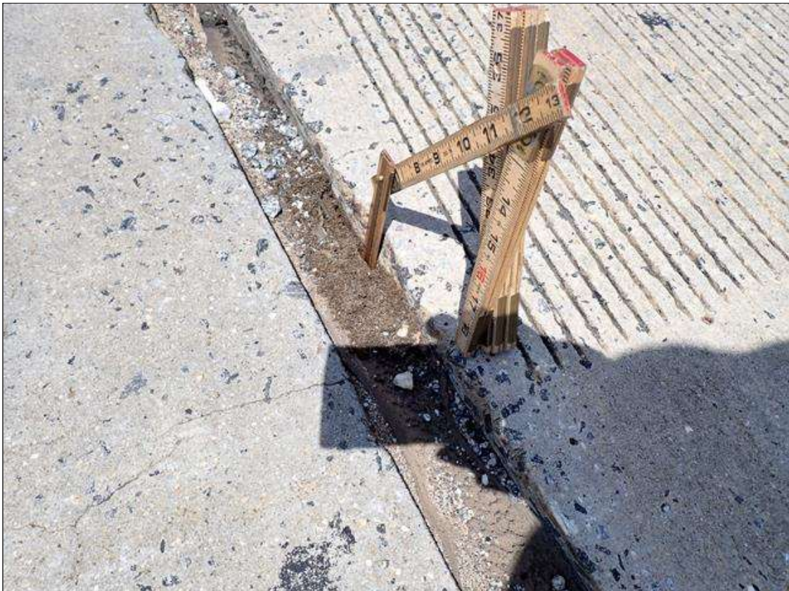
Span 1 Expansion Joint at End Bent 1: along the length of the joint, seal deteriorated/torn and adhesion loss (up to full length x full depth)
