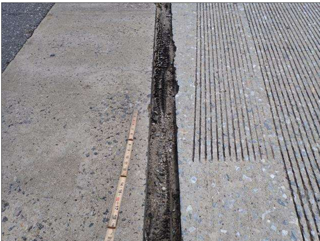
Span 2 Expansion Joint at End Bent 2: along the length of the joint, seal deteriorated/torn and adhesion loss (up to full length x full depth)
