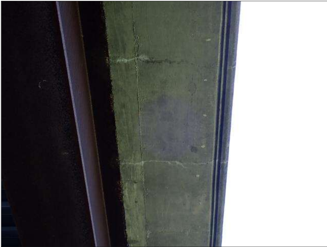
Span 2 Deck: underside of deck, both overhangs, transverse cracks (up to 1/32 inch x full width) some with efflorescence
