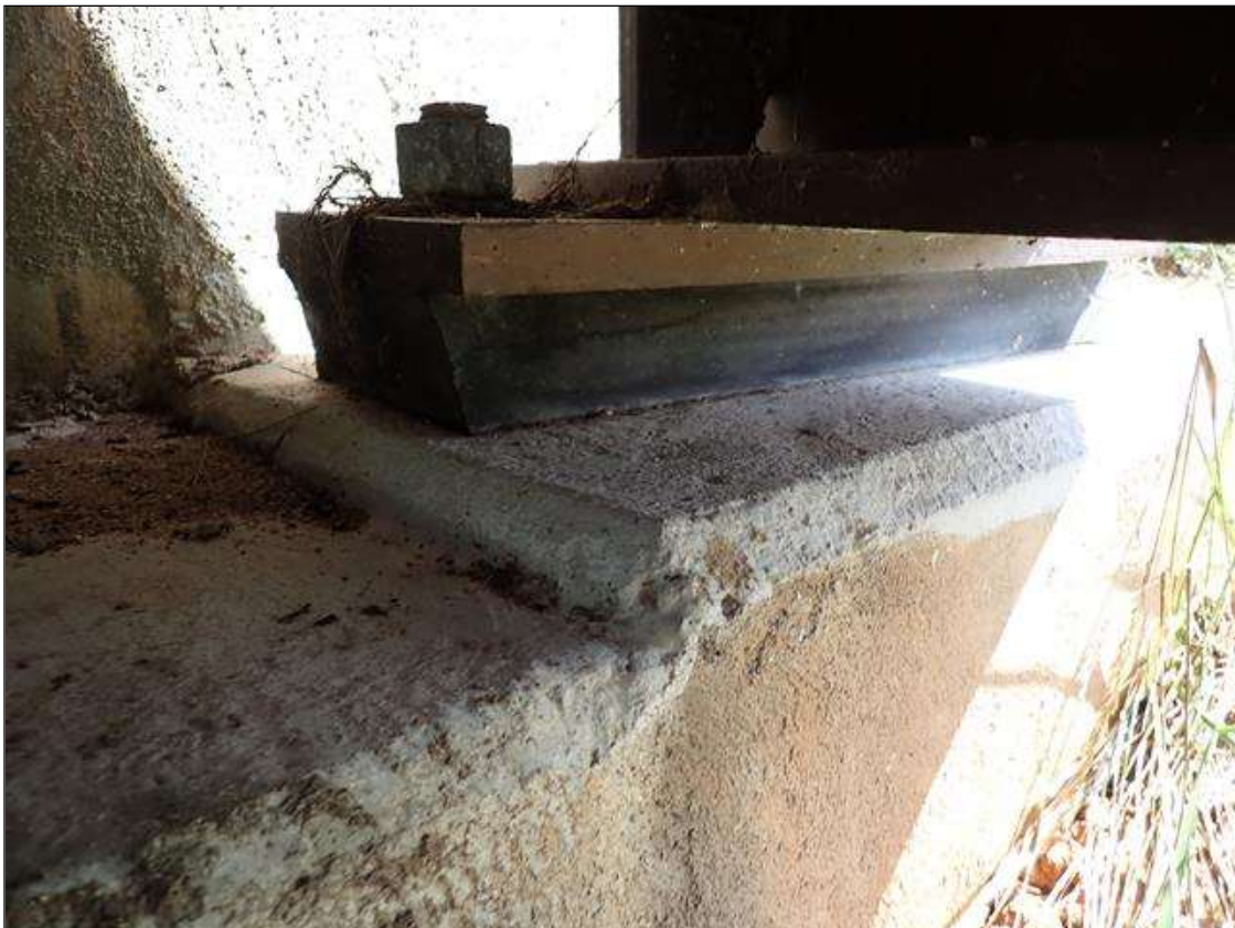
end bearing assembly
