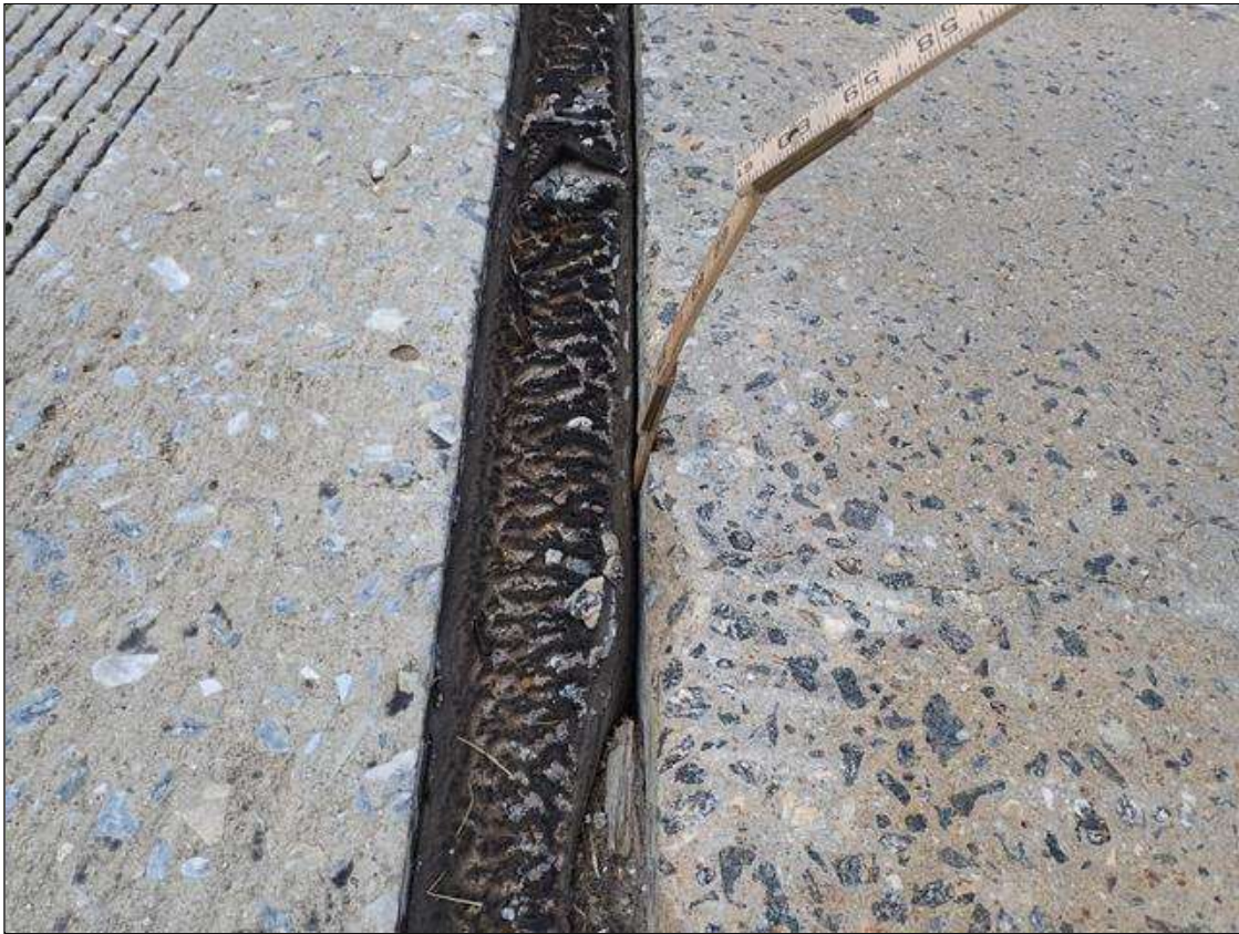
Span 2 Expansion Joint at End Bent 2: along the length of the joint, seal deteriorated/ torn and adhesion loss (up to full length x full depth)
