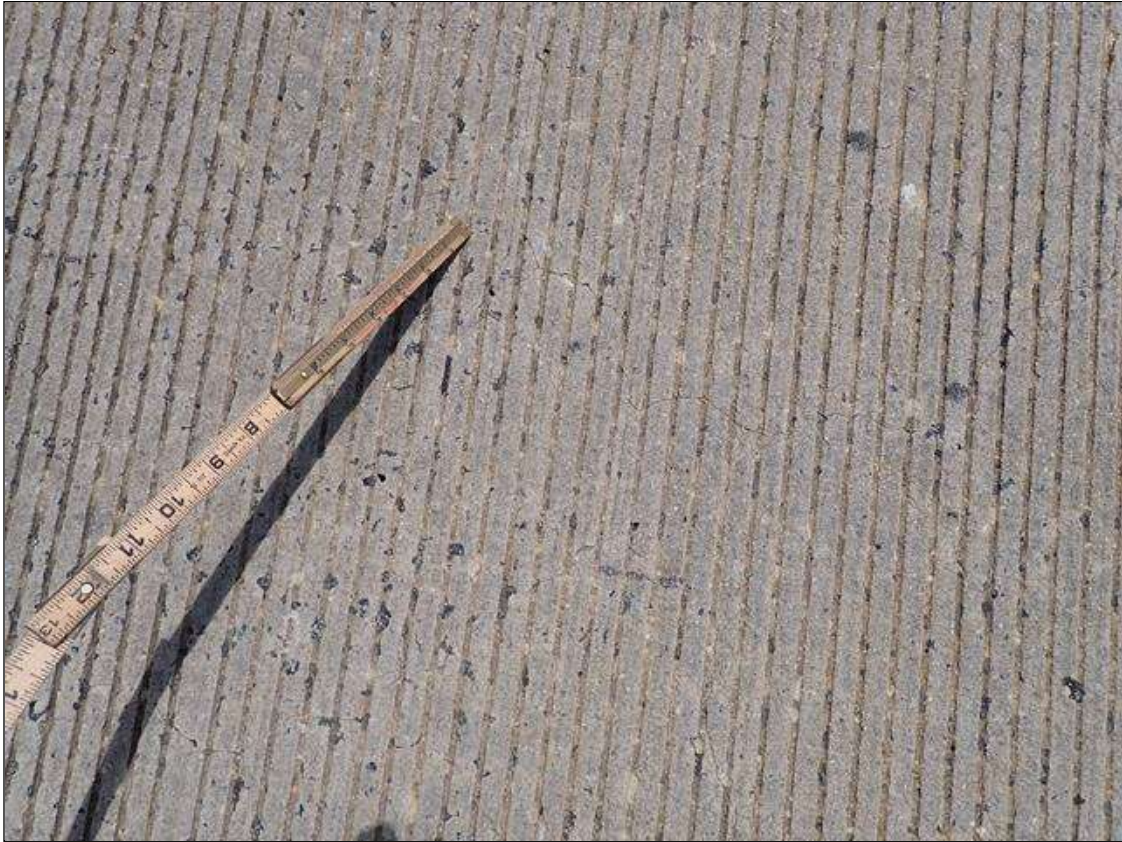
Span 1 Deck: throughout topside of deck, map cracks (hairline) and transverse/longitudinal cracks (up to 1/32 inch x 12 foot) at random
