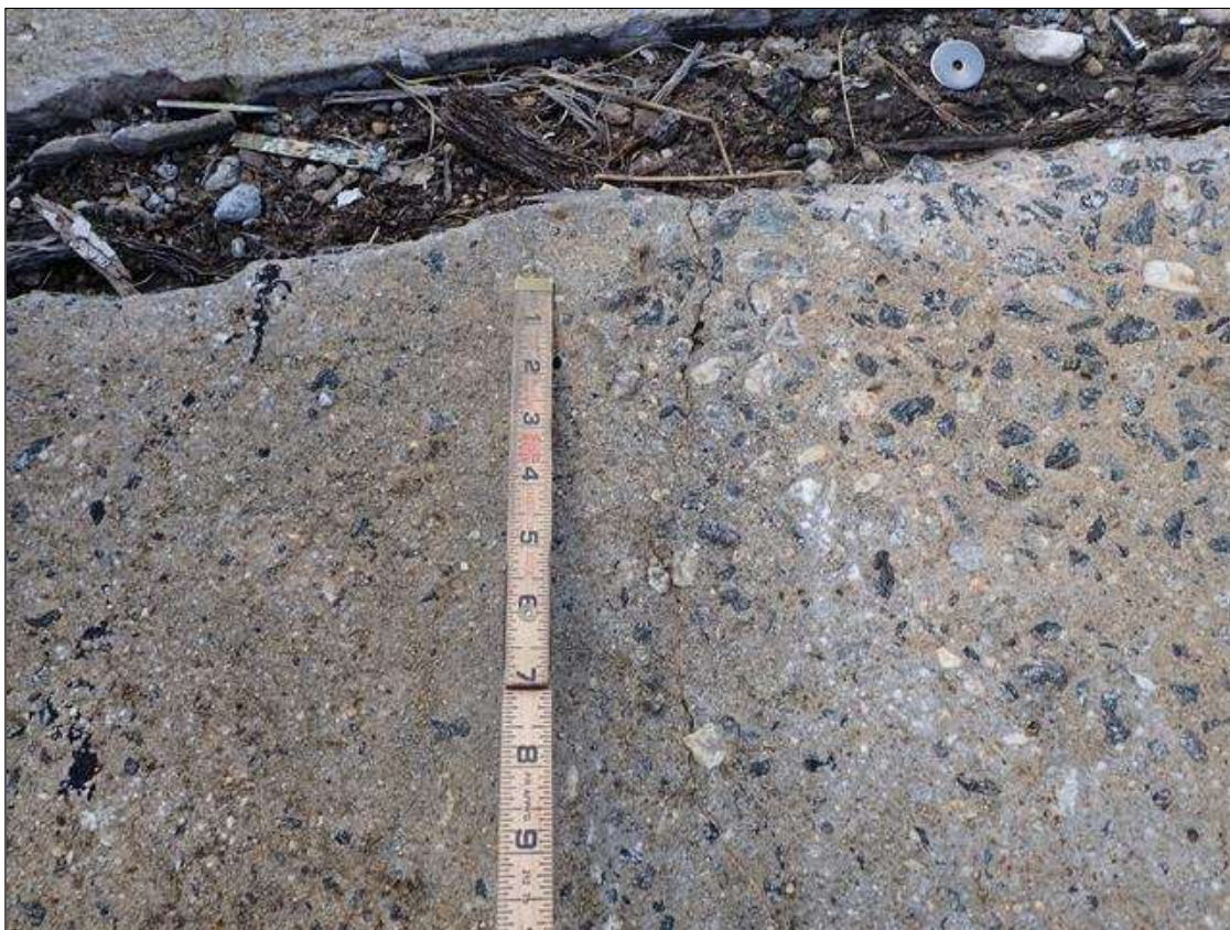
Approach 2 : SCATTERED LONGITUDINAL CRACKS THROUGH OUT [UP TO FULL WIDTH X 1/32 INCH]
