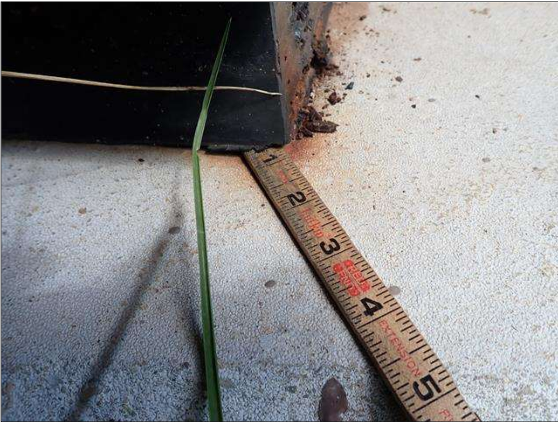
Span 1 Far Bearing 6: (PAR) east face, bulging (up to 1/8 inch high) with tear (10 inch x 1/4 inch wide) exposing steel plate; steel plate, rust scale; southeast corner, loss of bearing (1 inch x 1.5 inch)
