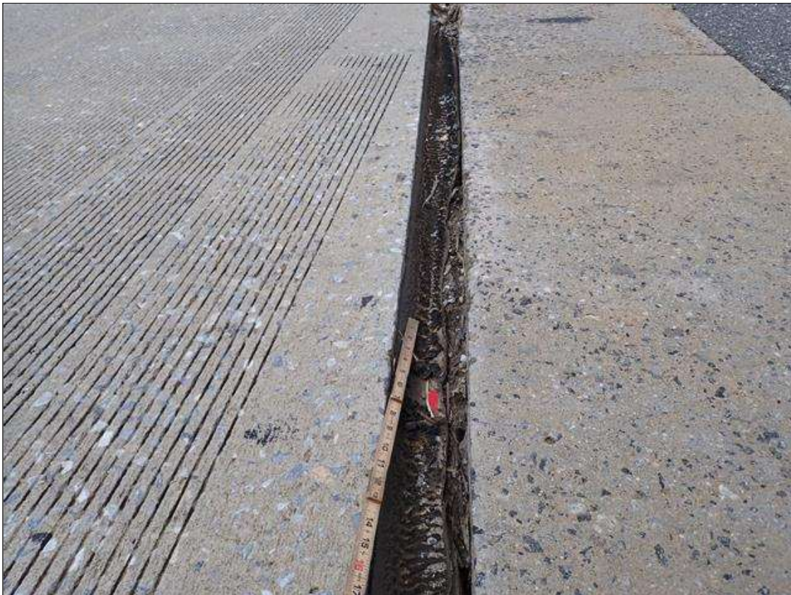
Span 2 Expansion Joint at End Bent 2: along the length of the joint, seal deteriorated/ torn and adhesion loss (up to full length x full depth)
