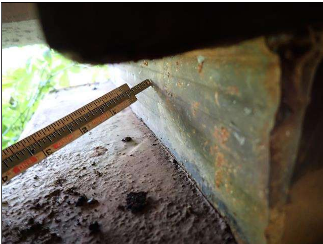
Span 1 Far Bearing 1: south face, bulging (up to 1/16 inch high)
