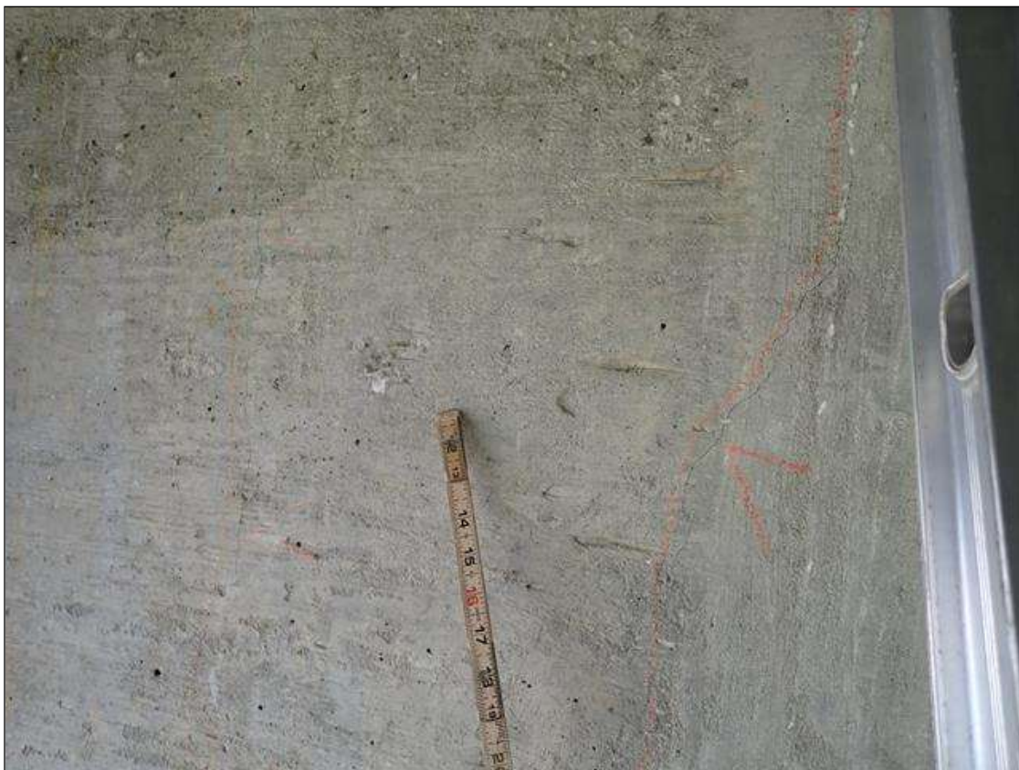
Bent 1 Cap 1: along the length of the cap, multiple vertical and diagonal cracks [up to full height x 1/32 inch] some extend across top
