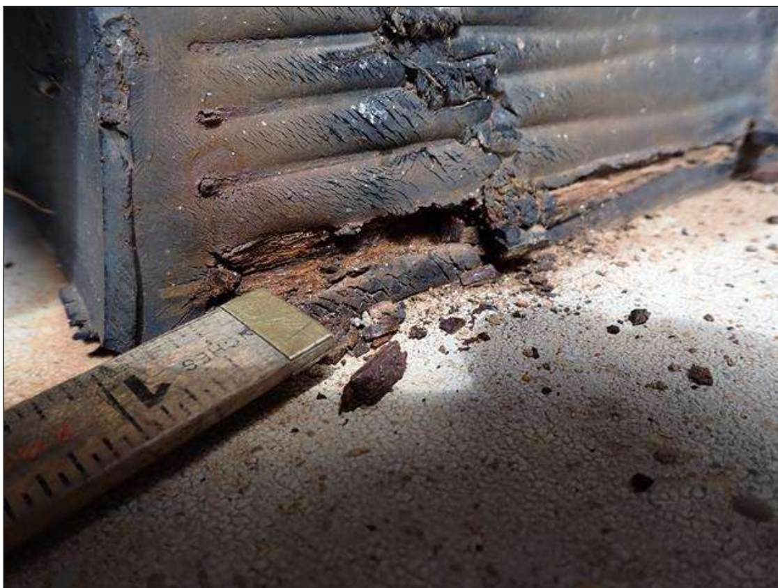
Span 1 Far Bearing 6: (PAR) east face, bulging (up to 1/8 inch high) with tear (10 inch x 1/4 inch wide) exposing steel plate; steel plate, rust scale; southeast corner, loss of bearing (1 inch x 1.5 inch)
