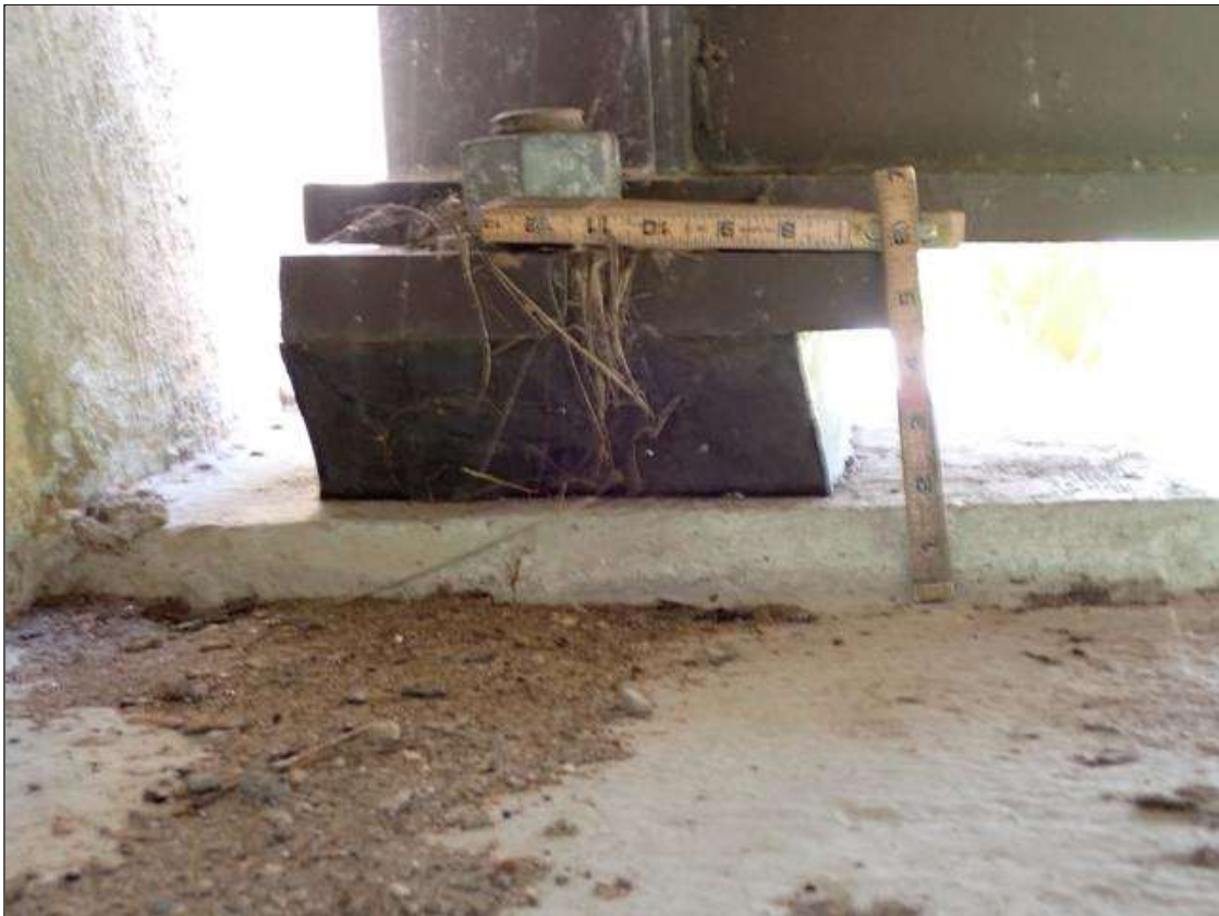
Span 1 Far Bearing 6: bearing is in expanded position (up to 1/2 inch); bearing pad, not flush with bearing plate (up to 1/8 inch)
