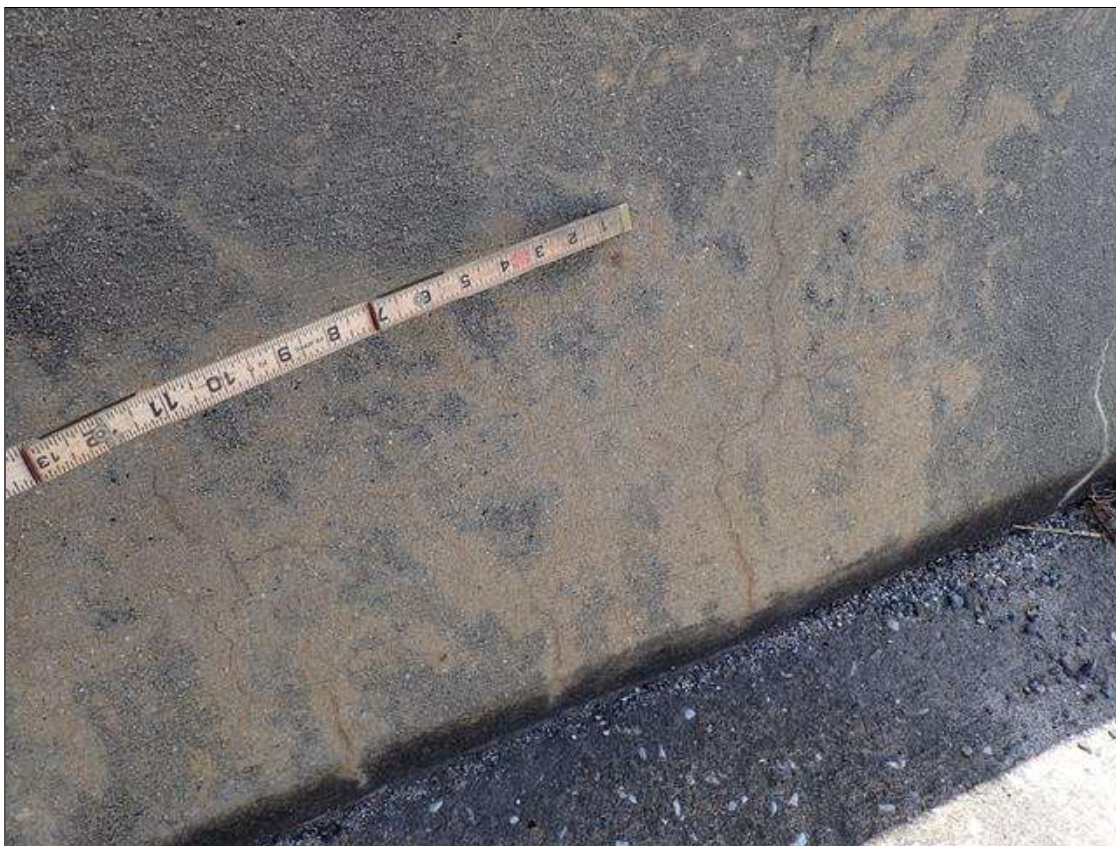
Span 2 Right Bridge Rail: along length of rail, map cracks [hairline] and multiple vertical cracks [up to full height x 1/32 inch], some wrap around, some with efflorescence
