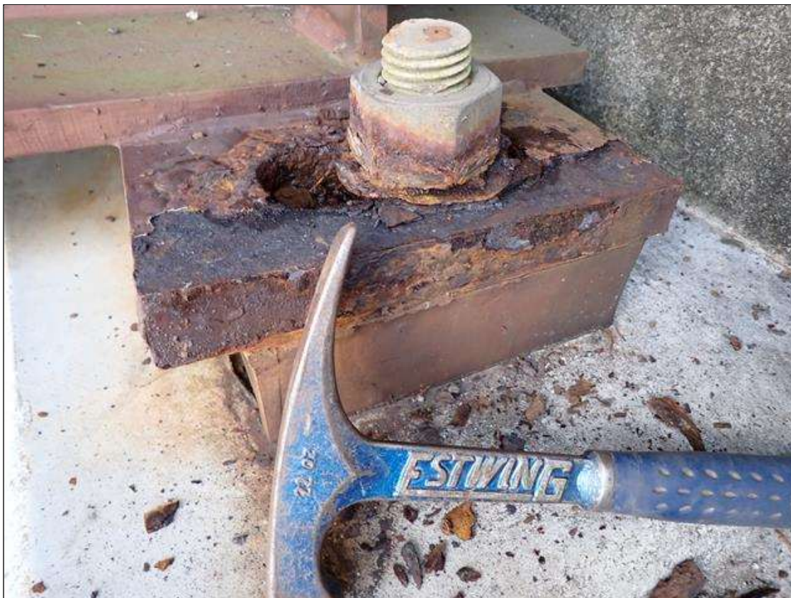
Span 1 Near Bearing 1: rust scale/corrosion with section loss (up to 1/16 inch loss)
