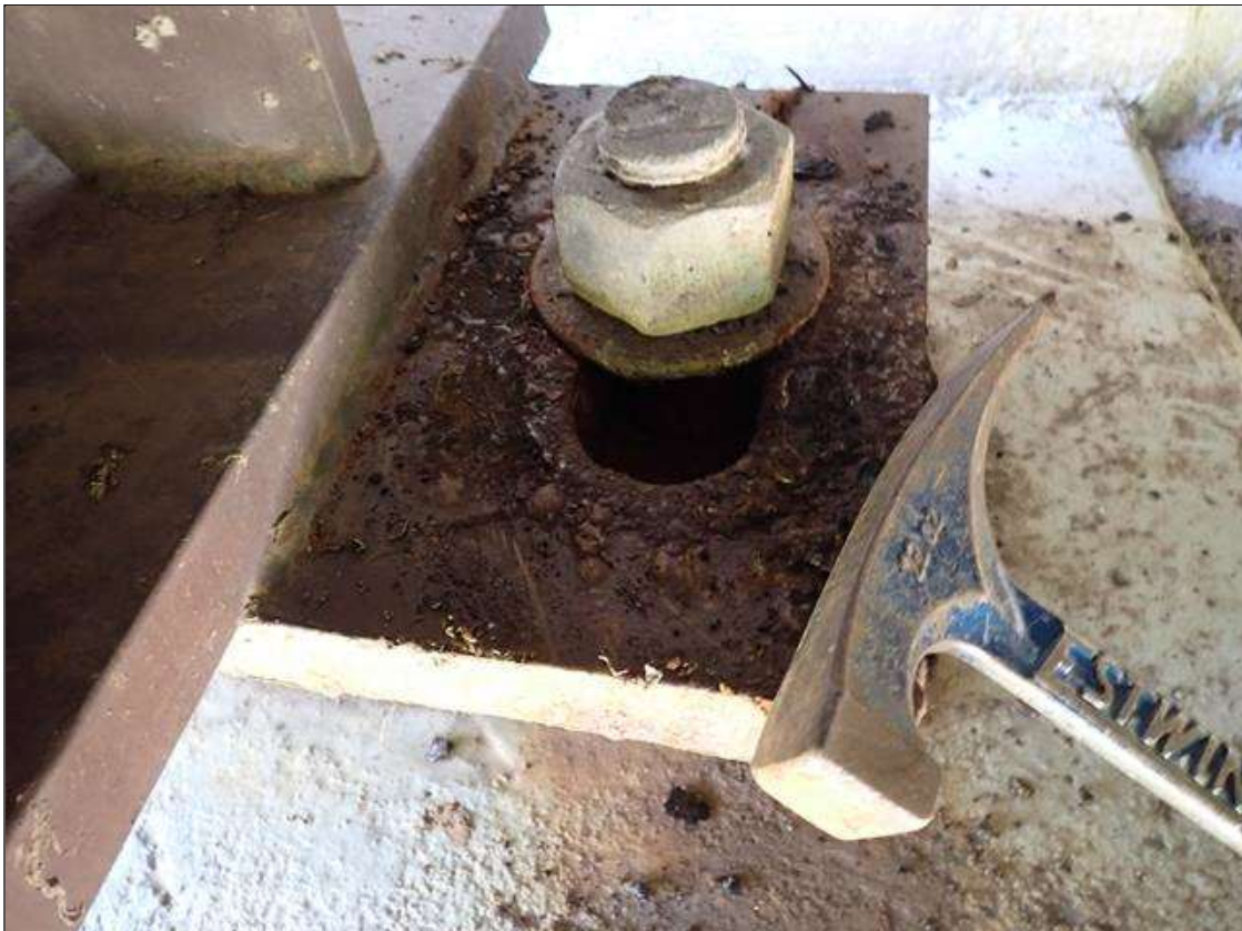
Span 1 Beam 1 - Far Bearing 1: rust scale (no measurable loss)
