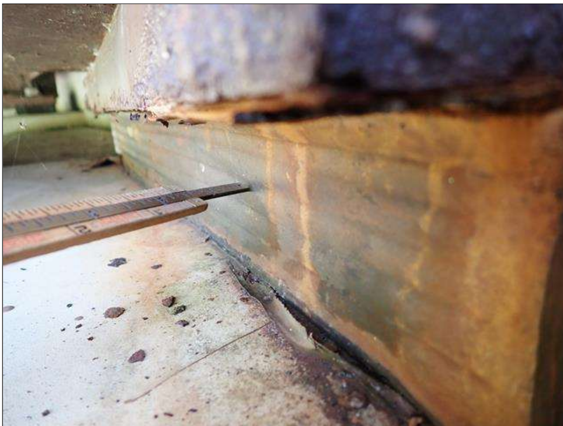
Span 1 Near Bearing 1: north face, bulging (up to 1/16 inch high)
