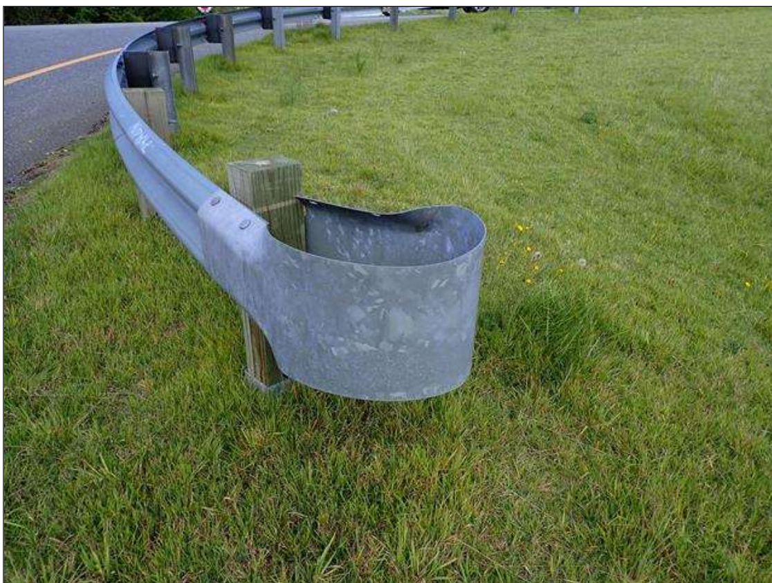
southeast guardrail termination
