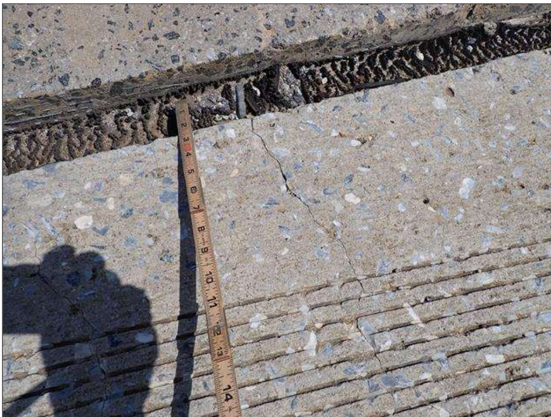
Span 2 Deck: throughout topside of deck, map cracks (hairline) and transverse/longitudinal cracks (up to 1/32 inch x 12 foot) at random
