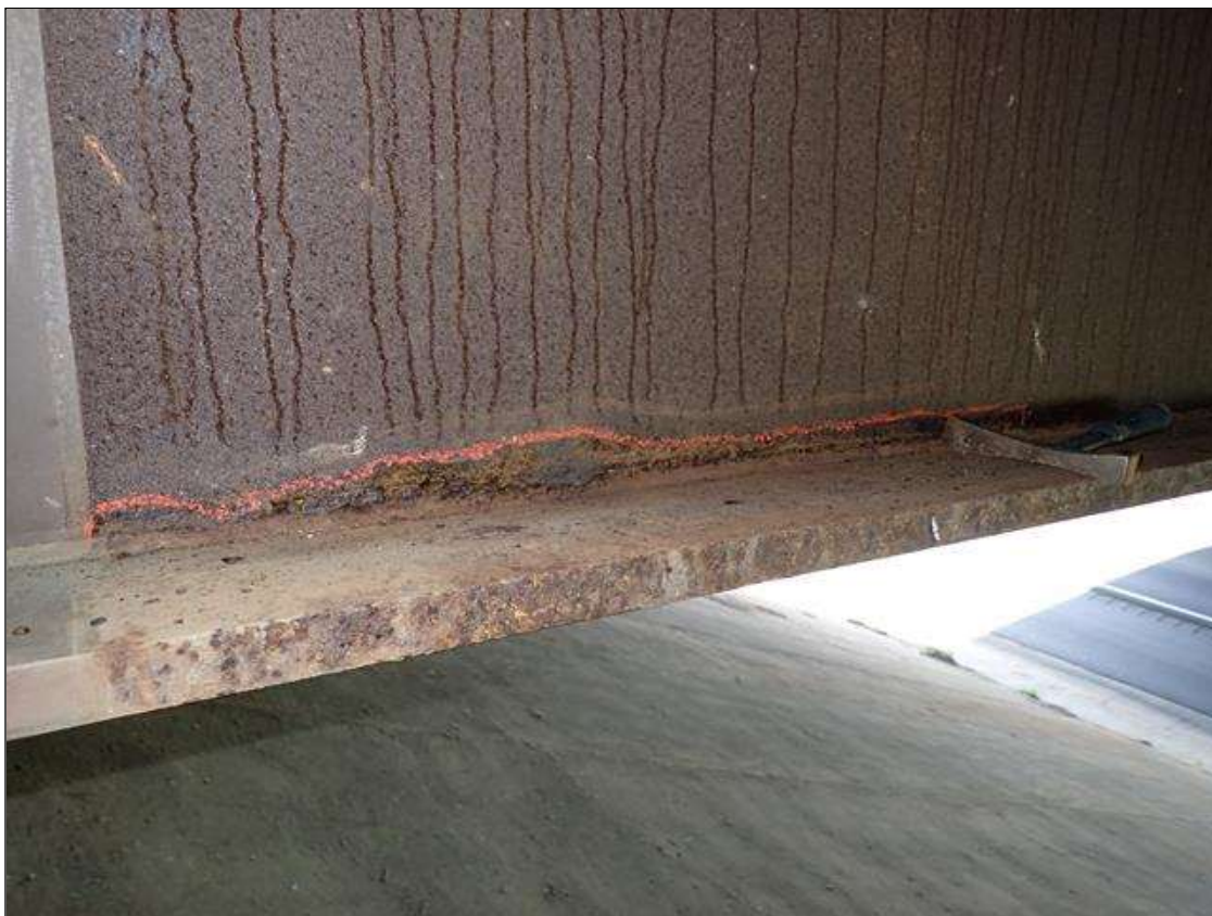
Span 1 Beam 2: (PAR) 6.5 foot from end bent 2, corrosion with section loss: lower web (3/8 inch average remaining x 34 inch x 2 inch); bottom flange, rust scale (9 foot)
