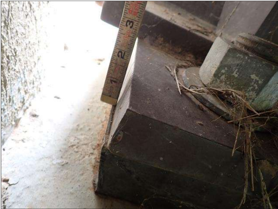
Span 1 Far Bearing 6: bearing is in expanded position (up to 1/2 inch); bearing pad, not flush with bearing plate (up to 1/8 inch)
