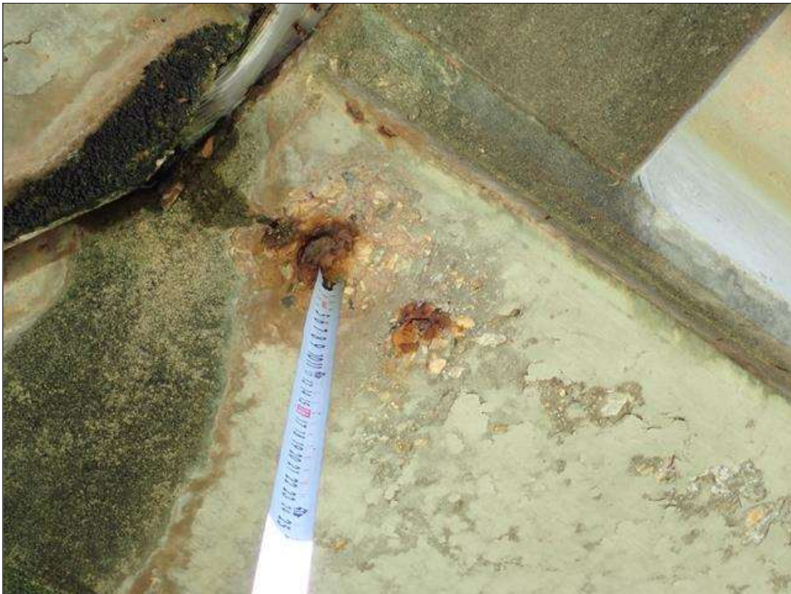
Span 2 Deck: (PAR) over bent 1, east overhang, spall (4 inch diameter x 1/2 inch deep) with exposed rusted rebar (approximately 25 percent loss)
