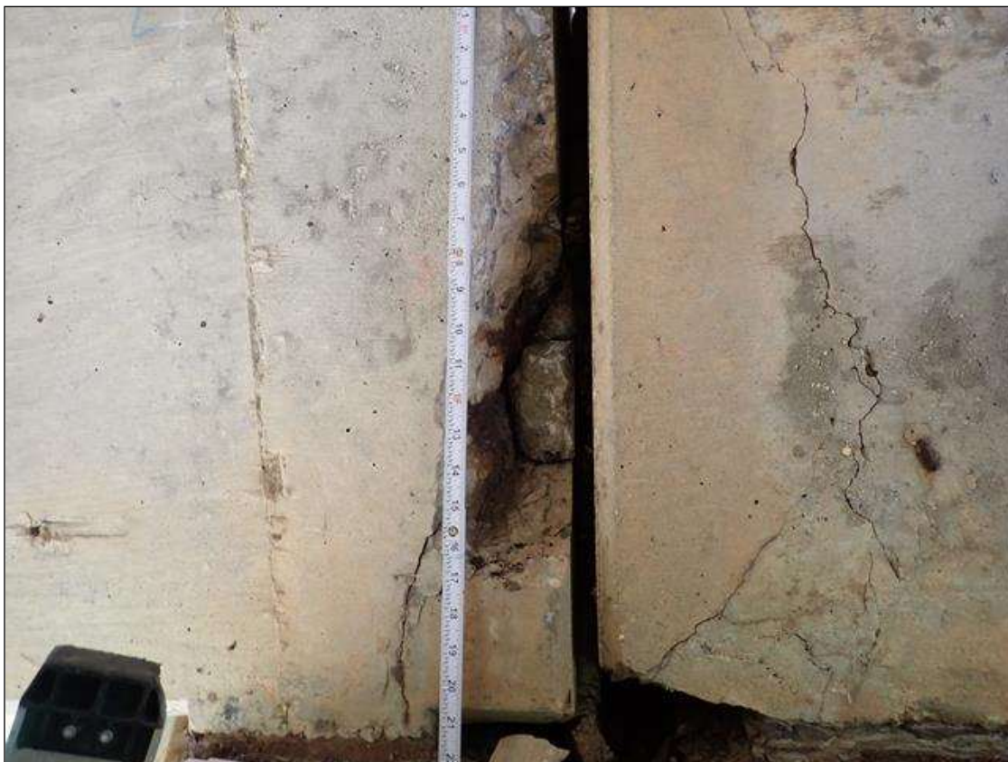
Span 5 Beam 3: (PAR) at bent 4, west face, spall/delamination (5 inch x 2 foot x 4 inch deep) with exposed rusted rebar (approximately 25 percent loss)
