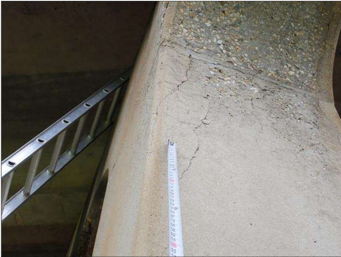
Bent 2 Pile 2: Southeast corner at corbel, delamination [54 inch x 20 inch] with cracks [up to 1/16 inch]
