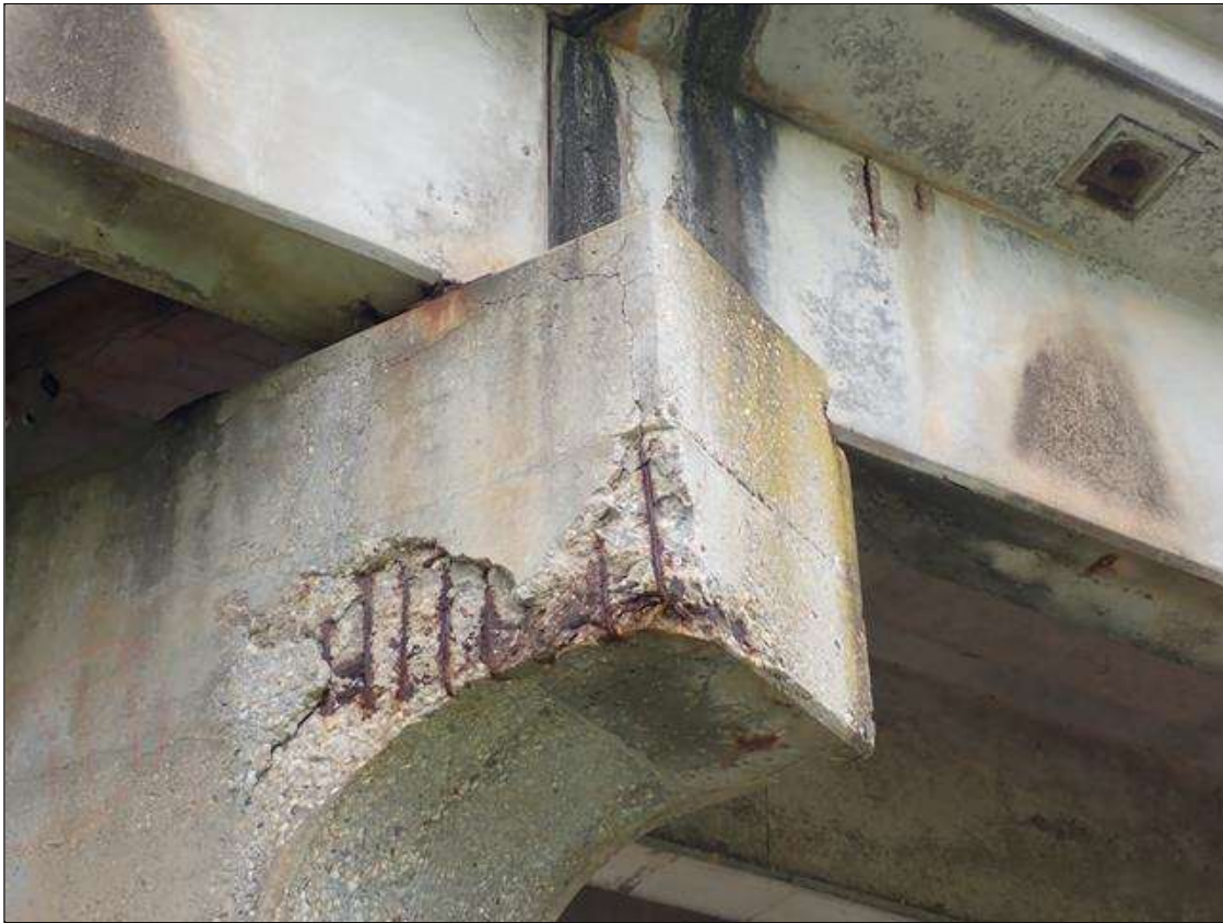
Bent 2 Cap 1: (PAR) South face at East end, spall/delamination [84 inch long x up to full height x up to 3 inch deep] with exposed rusted rebar and stirrups [rebar and stirrups with approximately 25 percent loss] and cracks [up to 1/8 inch]
