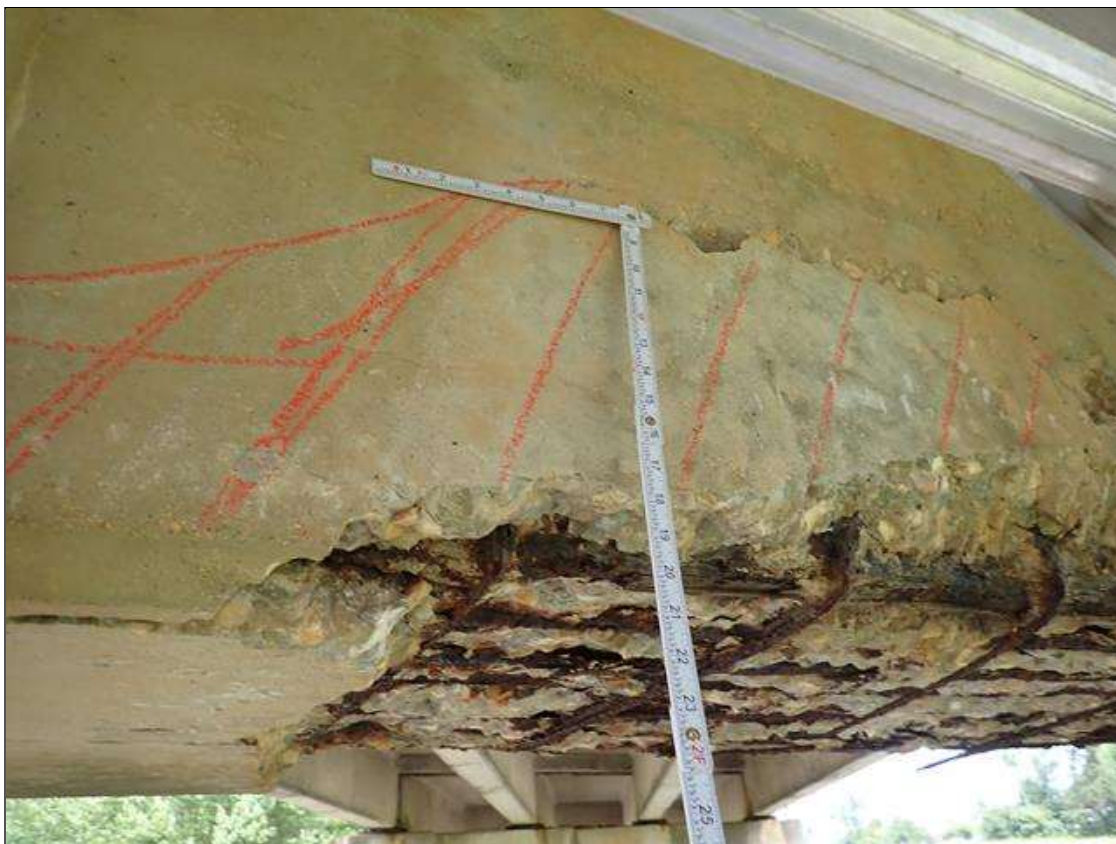
Bent 2 Cap 1: (PAR) underside of cap between columns, spall/delamination [14 foot long x full width x up to 4 inch deep] that extends onto south face [13 inch] with exposed rusted rebar and stirrups [rebars with approximately 25 percent loss; stirrups up to 100 percent loss]
