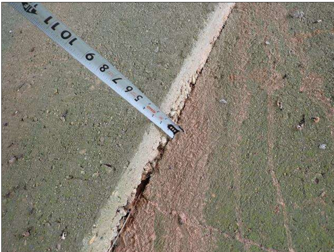
end bent 1 slope protection below bay 2, section misaligned/settled (up to 2 inch)
