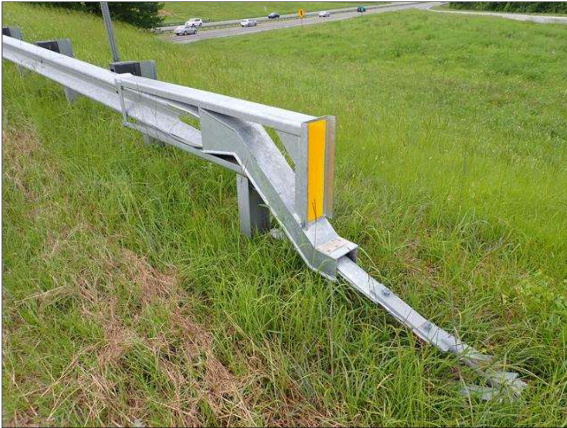
northwest guardrail termination
