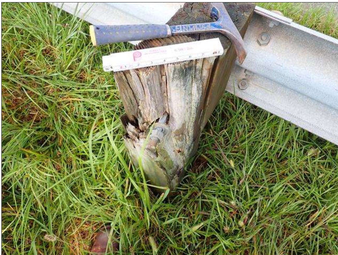
(PAR) northeast guardrail, 3rd and 12th timber posts from end bent 2, decay/section loss (up to full width x full height x full depth)
