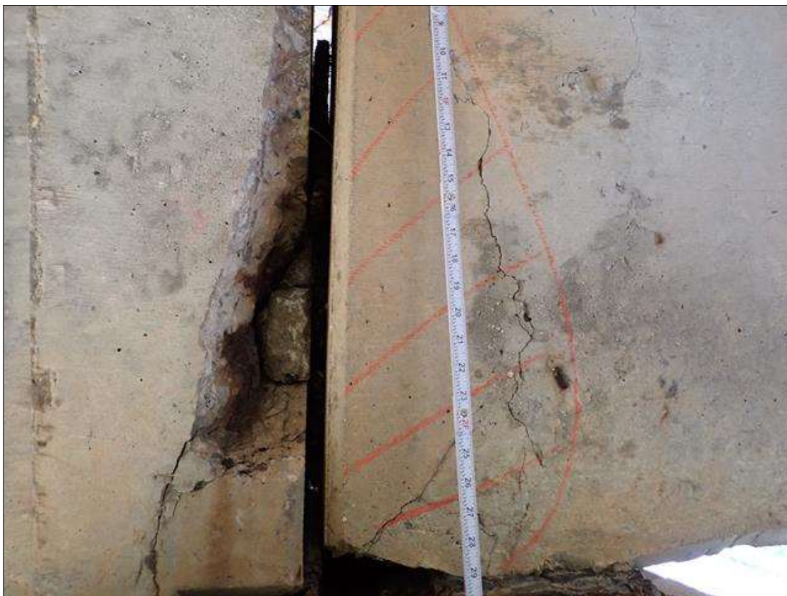
Span 4 Beam 3: SPAN 4 BEAM 3 WEST FACE OVER BENT 4. HAS A AREA THAT IS CRACKED (UP TO 1/16 INCH) AND DELAMINATED. AREA IS: (11 INCH X 31 INCH)
