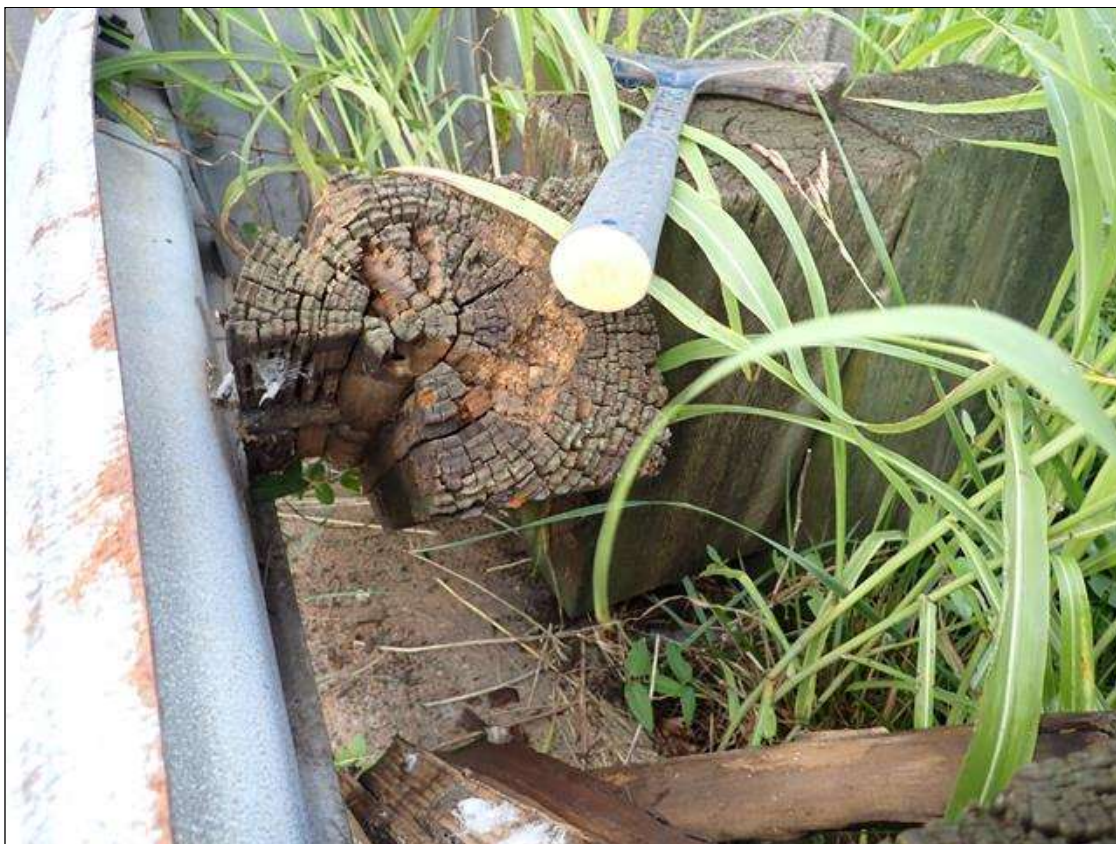
(PAR) northwest guardrail, 1st timber spacer from end bent 2, decay/section loss (full height x 3 inch x 3 inch deep)
