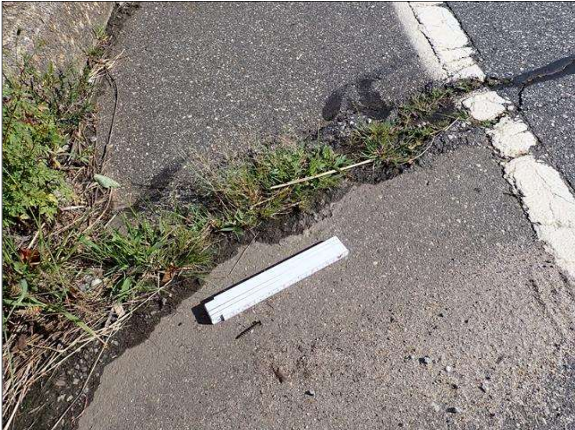
Span 2 Wearing Surface: over bent 2, partially sealed transverse crack (1/8 inch x full width) with edge spalling (up to 3 foot x 5 inch x 1/2 inch deep) with vegetation growth
