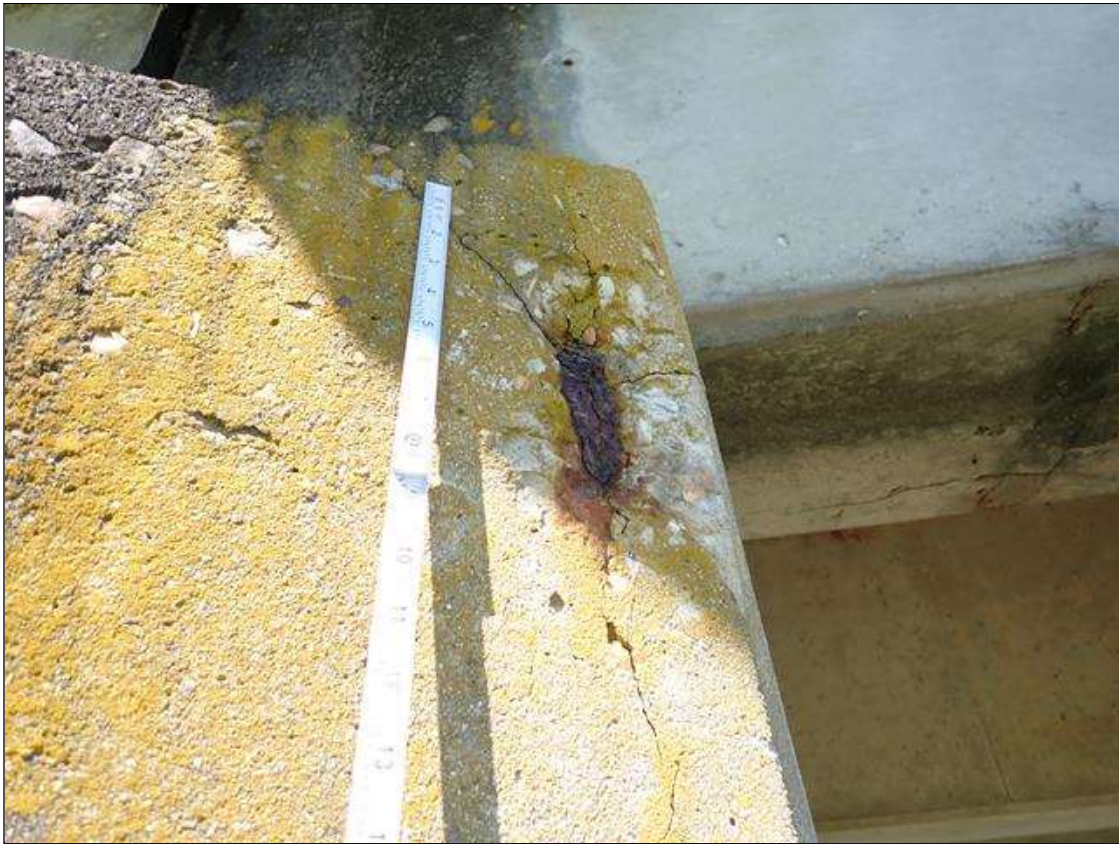
Bent 1 Cap 1: (PAR) east face, spall/delamination (12 inch x 6 inch x 1 inch deep) with exposed rusted rebar (approximately 25 percent loss)
