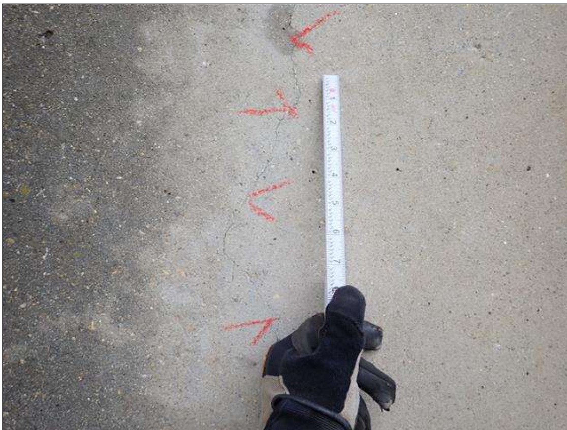
Bent 3 Pile 2: UP TO 8 FOOT X UP TO 1/32 INCH VERTICAL CRACKS, AT RANDOM THROUGHOUT.
