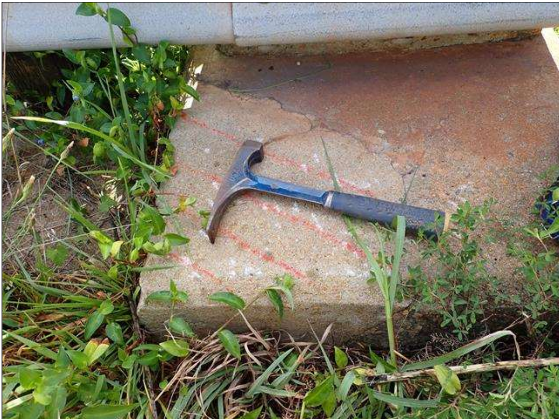
Span 5 Right Bridge Rail: at far end of right sidewalk, partially sound patch [14 inch x 16 inch]
