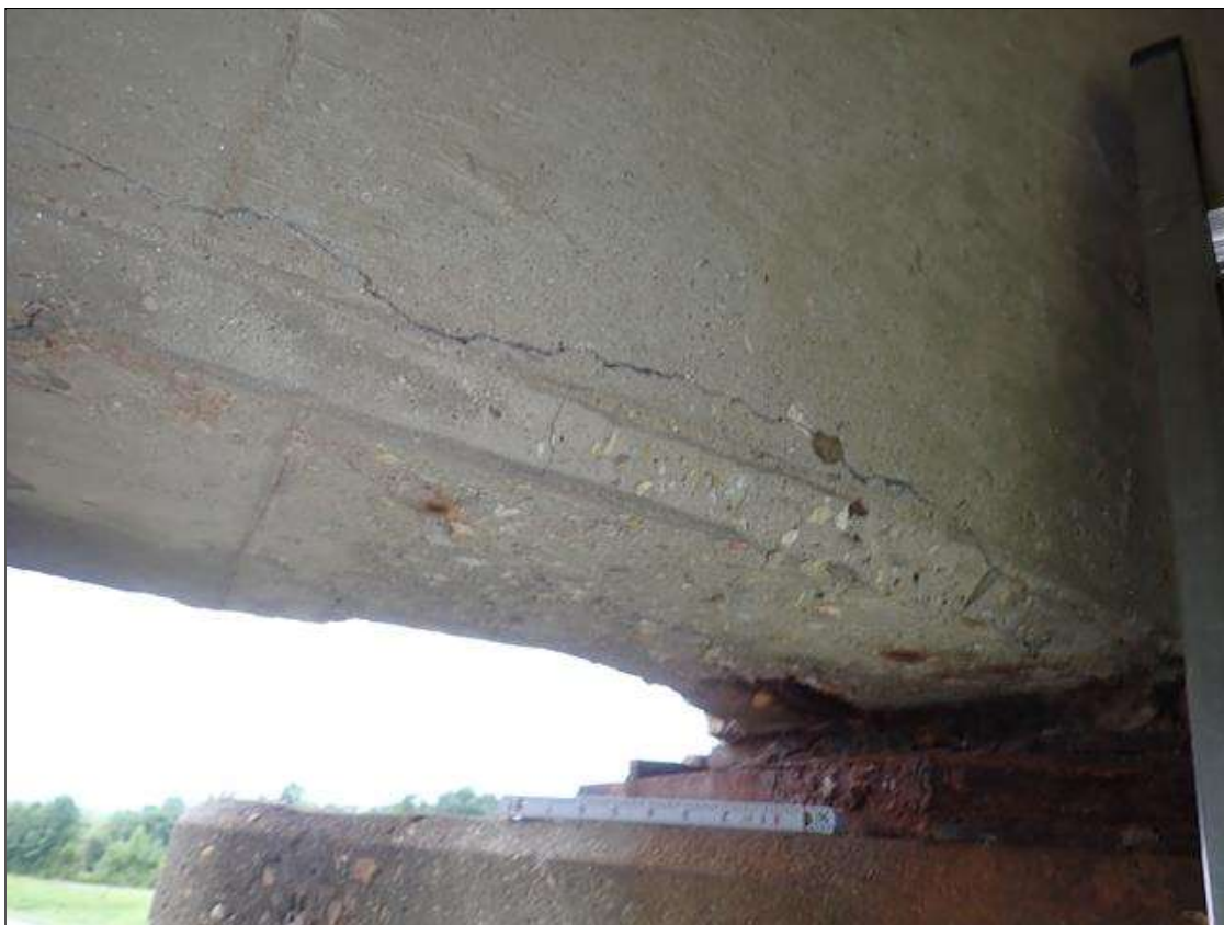
Span 2 Beam 1: (PAR) at bent 2, west face and underside, multiple spalls/delaminations (2 foot x 32 inch x 2.5 inch deep) with exposed rusted rebar (approximately 25 percent loss) and cracks (up to 1/8 inch)
