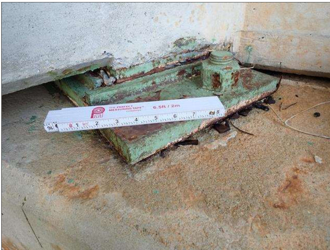
Span 1 Near Bearing 1: SURFACE RUST
