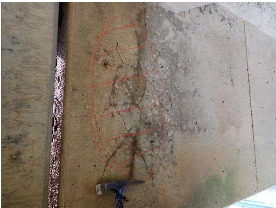
Span 4 Beam 4: West face over bent 4, delamination/spall [1 foot x 2 foot] with map cracks (up to 1/32 inch)
