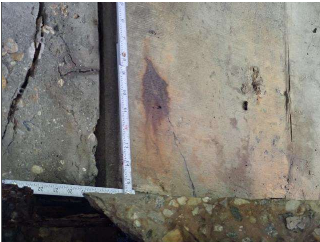
Span 2 Beam 1: (PAR) East face at near end, vertical crack [10 inch x 1/32 inch] with rust stain
