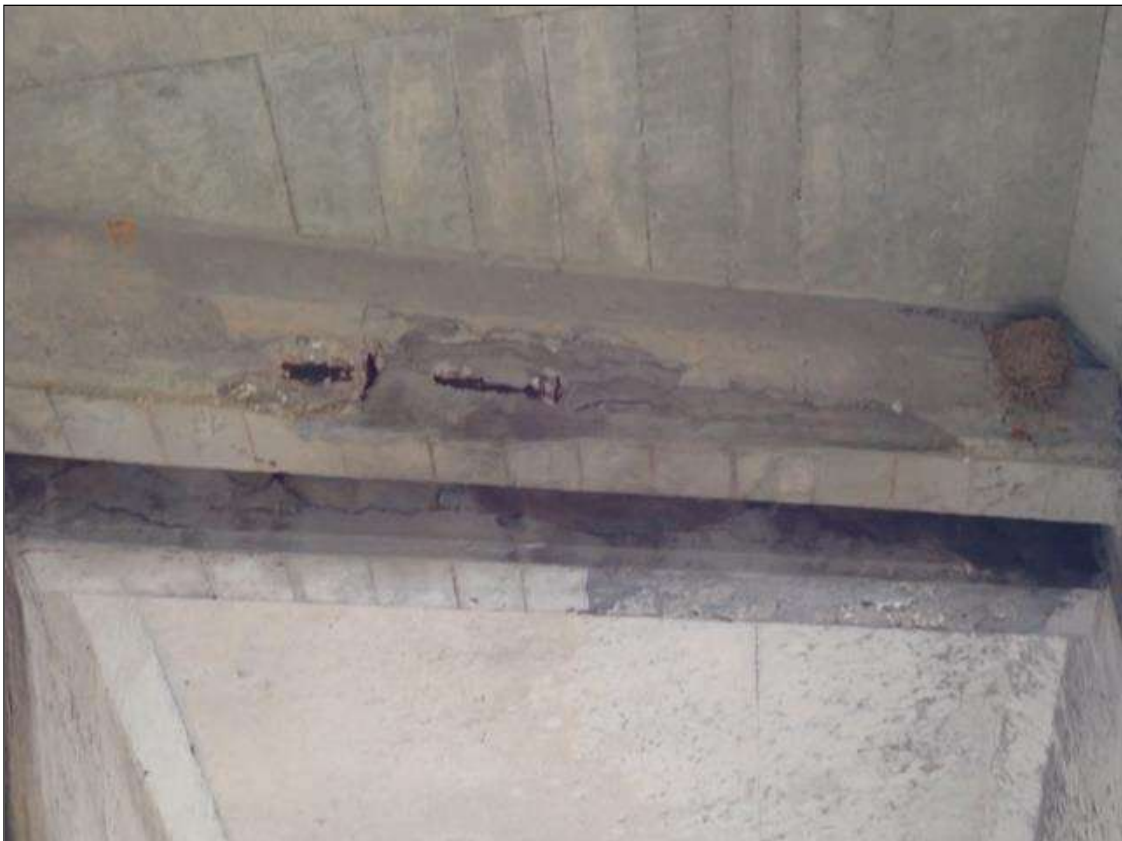
Span 5 Beam 1: 4 FOOT X 10 INCH X 1/2 INCH DEEP FAILED PATCH WITH EXPOSED REINFORCING, IN BENT 4 DIAPHRAGM, BAY 1.
