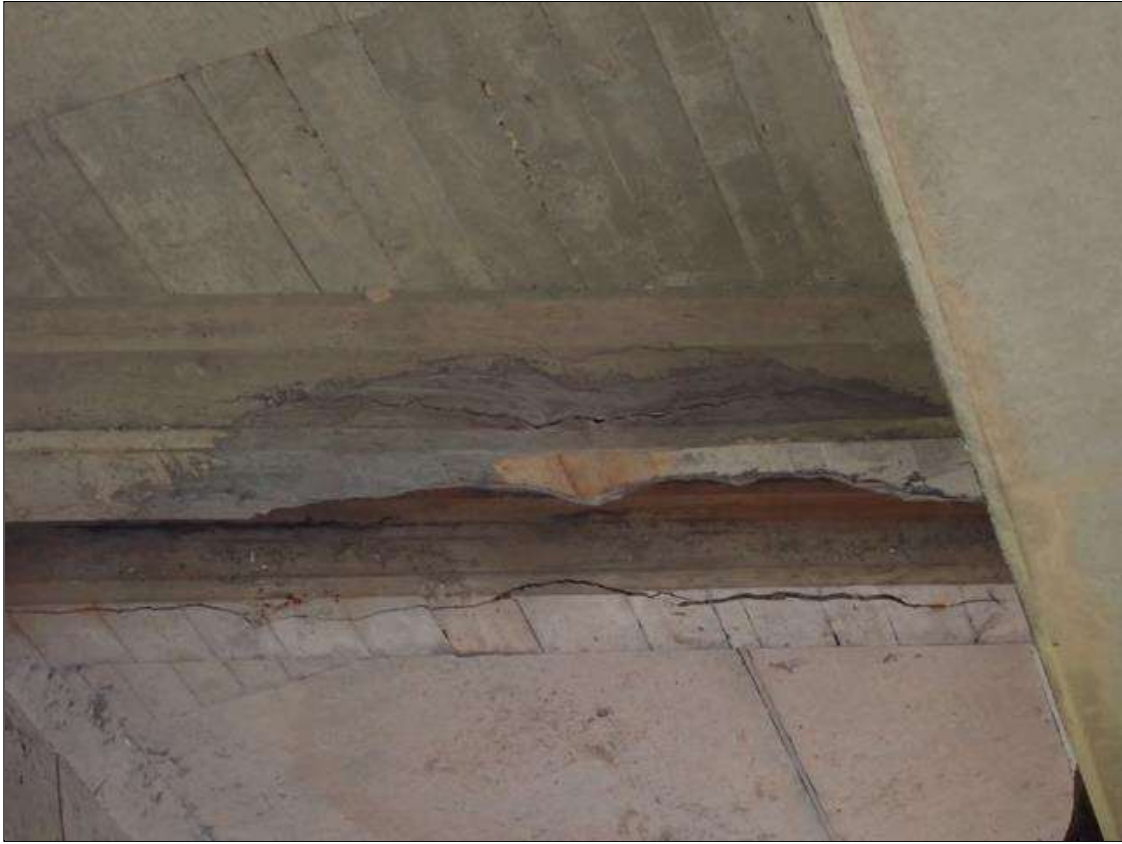
Span 5 Beam 3: 4 FOOT X 8 INCH X 8 INCH CRACKED PATCHED AREA, IN BENT 4 DIAPHRAGM, BAY 3.
