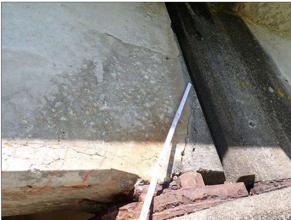
Span 1 Beam 4: (PAR) at bent 1, west and east faces and underside, multiple spalls/delaminations (up to 8 inch x 12 inch x 1/2 inch deep) with exposed rusted rebar (approximately 25 percent loss) and cracks (up to 1/8 inch)
