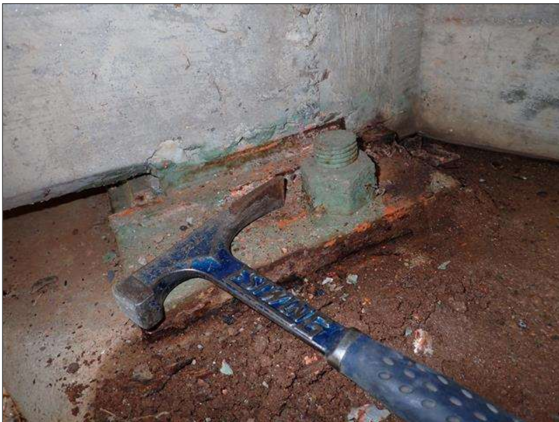
Span 5 Far Bearing 1: rust scale
