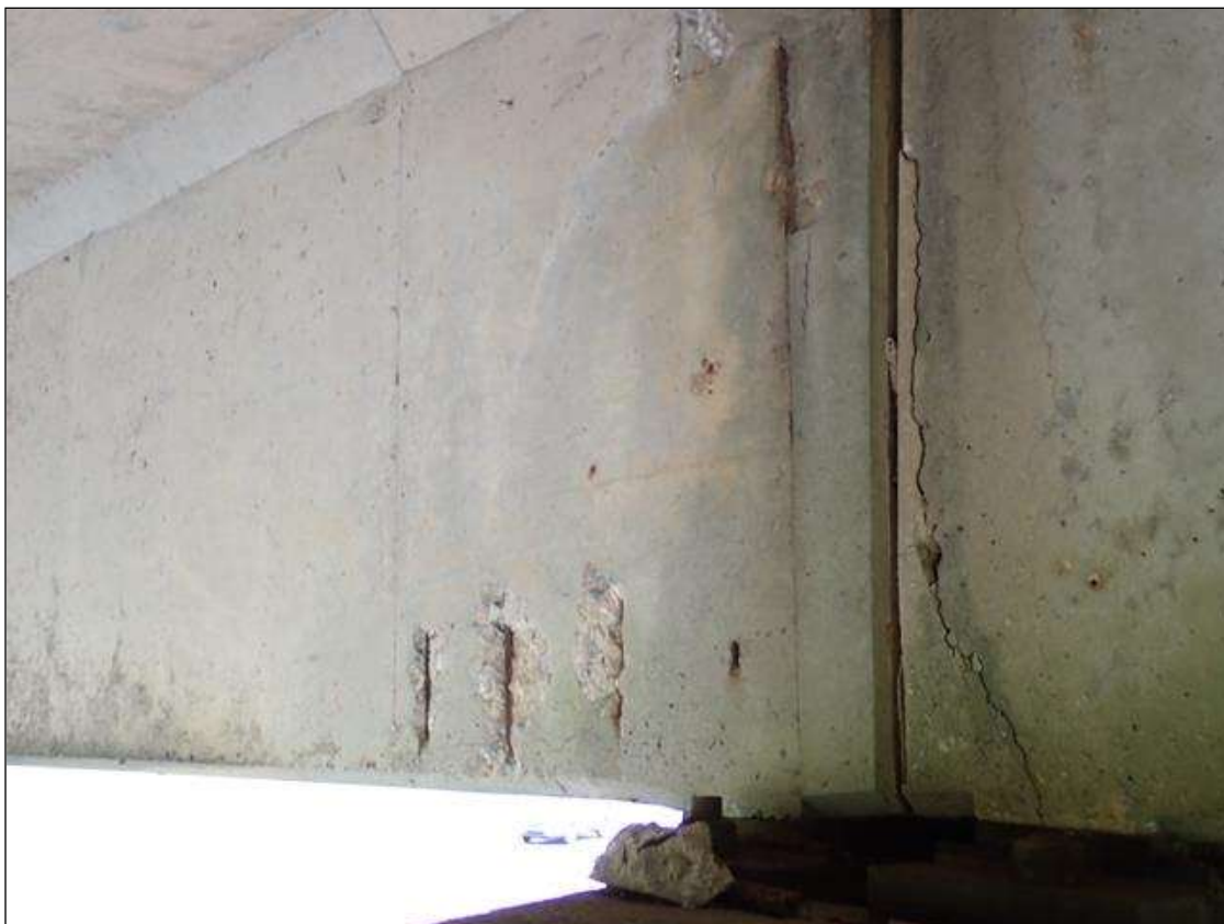
Span 3 Beam 2: (4)- UP TO 3 INCH X 12 INCH X 1 INCH SPALLS WITH EXPOSED REINFORCING, WEST FACE, AT BENT 2.
