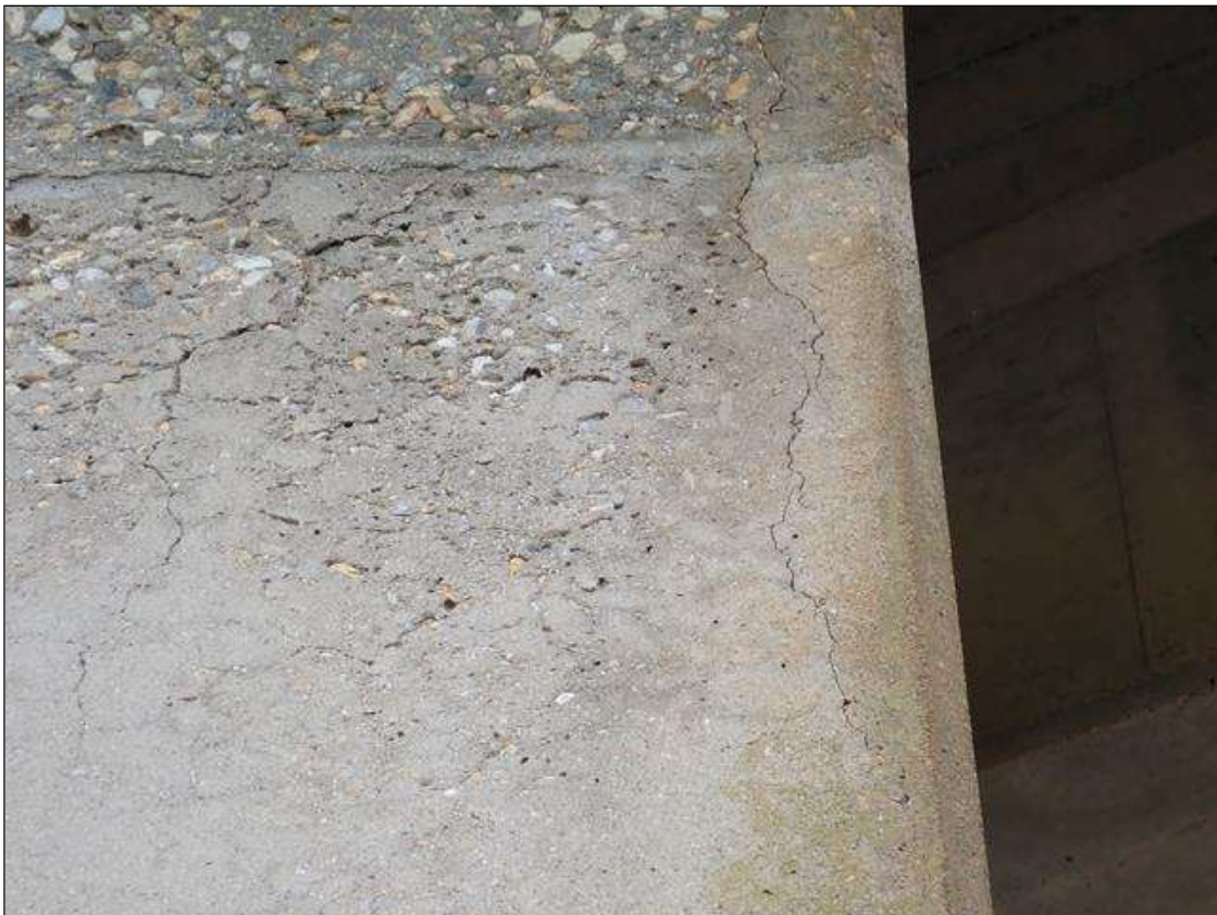
Bent 2 Pile 2: UP TO 5 FOOT X UP TO 1/16 INCH VERTICAL CRACKS, AT RANDOM THROUGHOUT, BEGINNING AT BOTTOM OF CAP.
