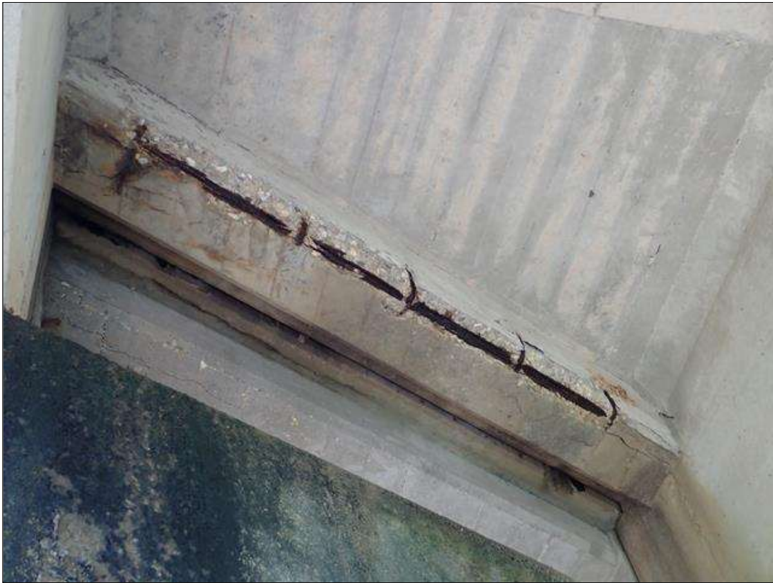
Span 2 Beam 3: (PAR) at bents 1 and 2, bay 3 end diaphragm, spalls/delaminations (up to full length x 8 inch x 1.5 deep) with exposed rusted rebar (approximately 25 percent loss)
