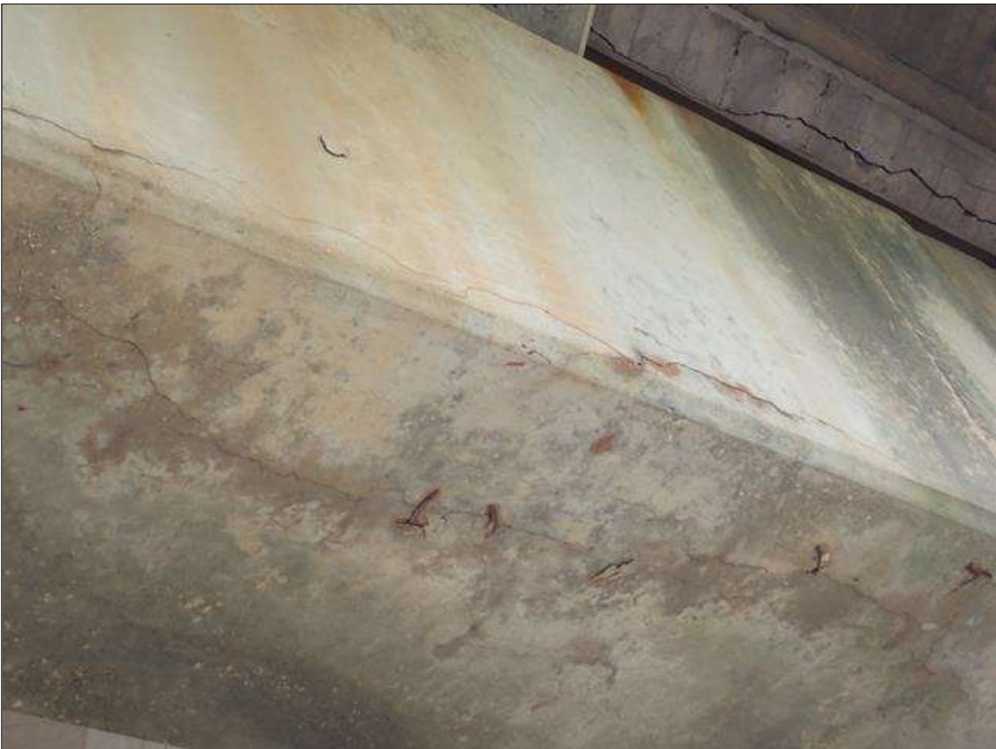
Bent 3 Cap 1: (PAR) BENT 3 CAP HAS SCATTERED CRACKS UP TO 1/16 INCH SOME WITH ADJACENT DELAMINATION (UP TO 7 FOOT X 1.5 FOOT) AND RUST STAINS.
