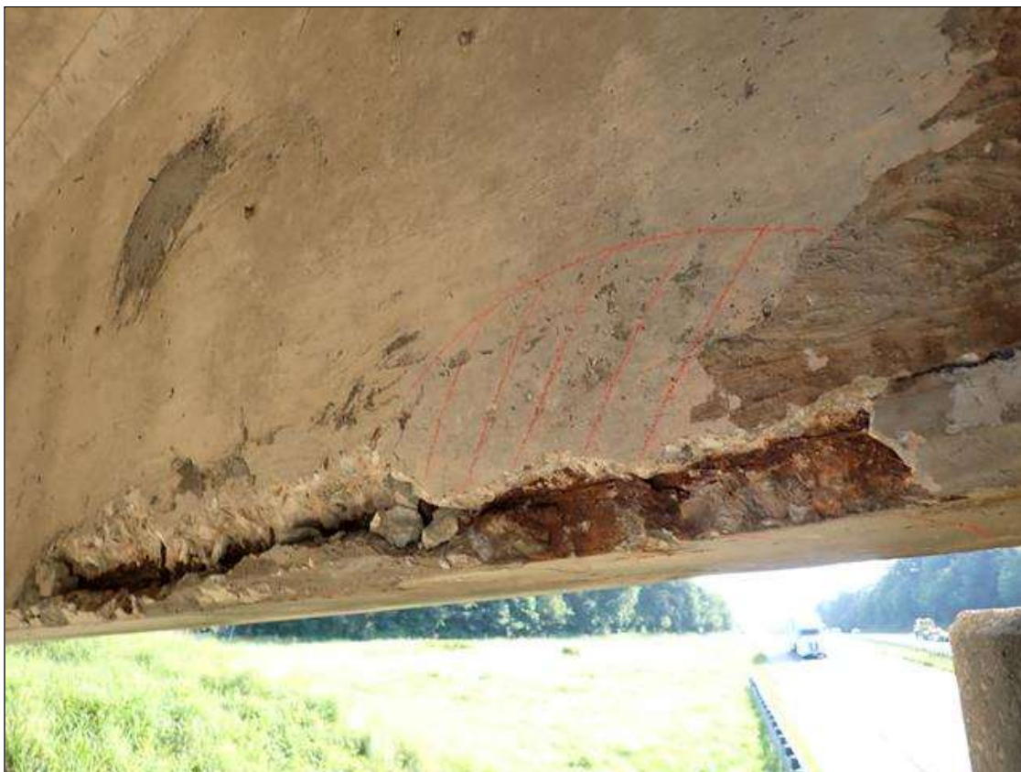
Span 5 Beam 4: (PAR) at bent 4, west face and underside, spall/delamination (6 foot x full width x up to 6 inch x 1.5 inch deep) with exposed rusted rebar (approximately 25 percent loss)
