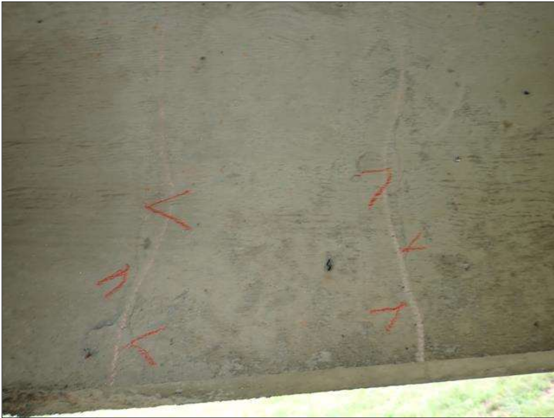
Span 2 Beam 4: TRANSVERSE AND WRAPAROUND CRACKS UP TO 1/64 INCH, AT RANDOM THROUGHOUT.
