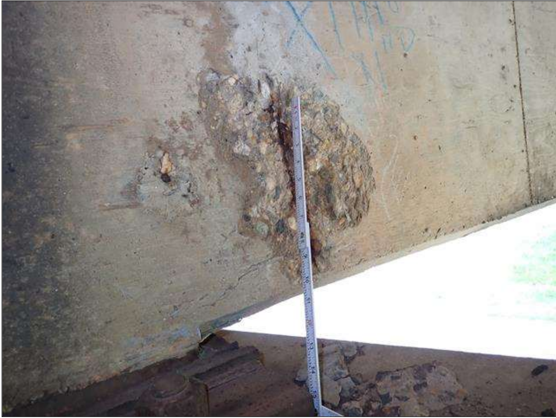
Span 3 Beam 3: (PAR) at bent 3, west face, spall/delamination (11 inch x 11 inch x 1/2 inch deep) with exposed rusted rebar (approximately 25 percent loss) and cracks (up to 1/32 inch)
