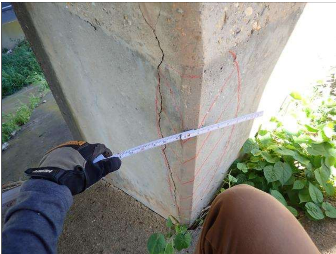
Bent 1 Pile 2: at Southwest corner, delamination [full height x 12 inch] with cracks (up to 1/8 inch)
