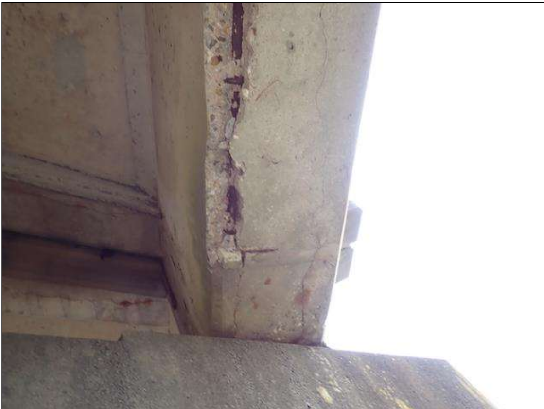
Span 4 Beam 1: (PAR) at bent 3, east face and underside, spalls/delaminations (up to 6 foot x 18 inch x 2 inch deep) with exposed rusted rebar (approximately 25 percent loss) and cracks (up to 1/16 inch)
