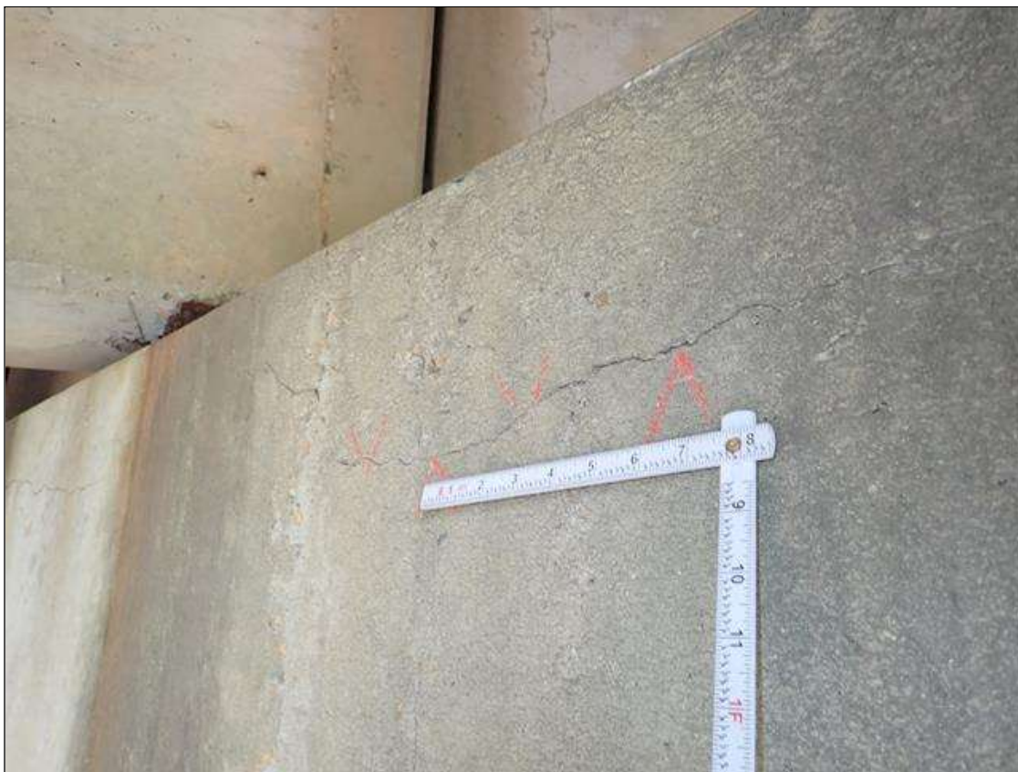
Bent 3 Cap 1: (PAR) BENT 3 CAP HAS SCATTERED CRACKS UP TO 1/16 INCH SOME WITH ADJACENT DELAMINATION (UP TO 7 FOOT X 1.5 FOOT) AND RUST STAINS.
