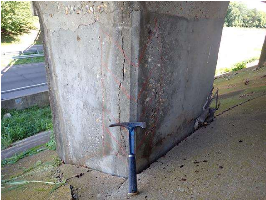
Bent 1 Pile 1: northwest, northeast and southwest corners, delaminations (up to full height x 16 inch) with cracks (up to 1/8 inch)
