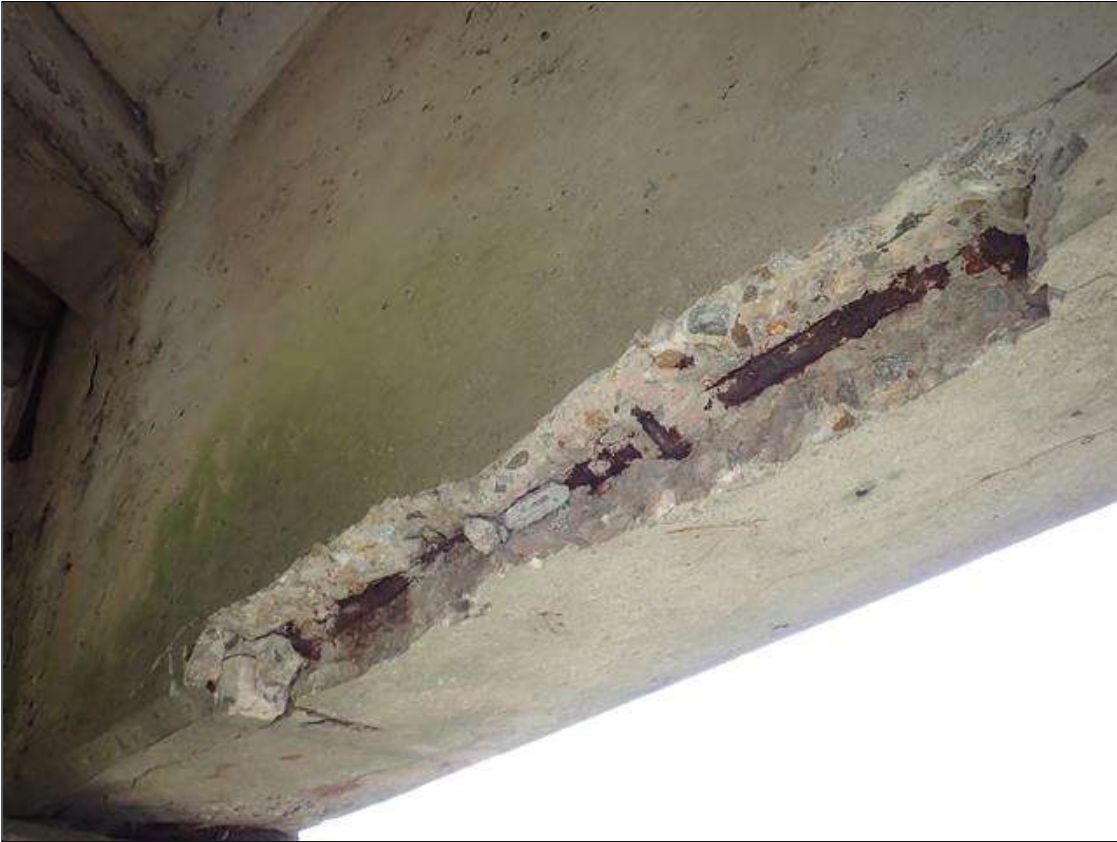
Span 4 Beam 1: (PAR) at bent 3, east face and underside, spalls/delaminations (up to 6 foot x 18 inch x 2 inch deep) with exposed rusted rebar (approximately 25 percent loss) and cracks (up to 1/16 inch)
