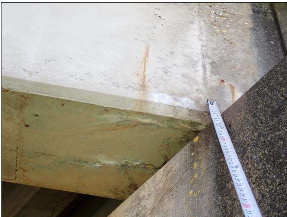
Span 2 Beam 1: (PAR) West face at near end, longitudinal crack [4 foot x 1/32 inch] and diagonal crack [full height x 1/32 inch] with rust stain and efflorescence
