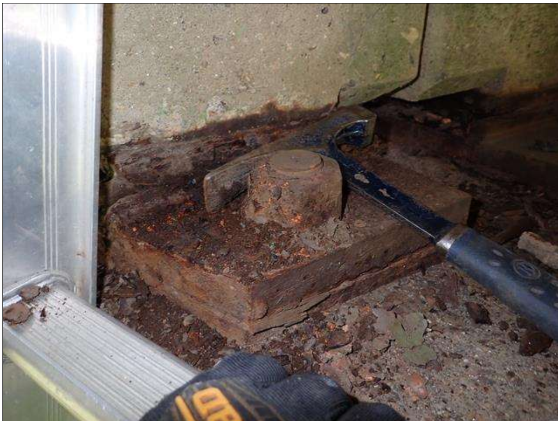
Span 2 Beam 1 - Far Bearing 1: corrosion with section loss [up to 1/8 inch loss]
