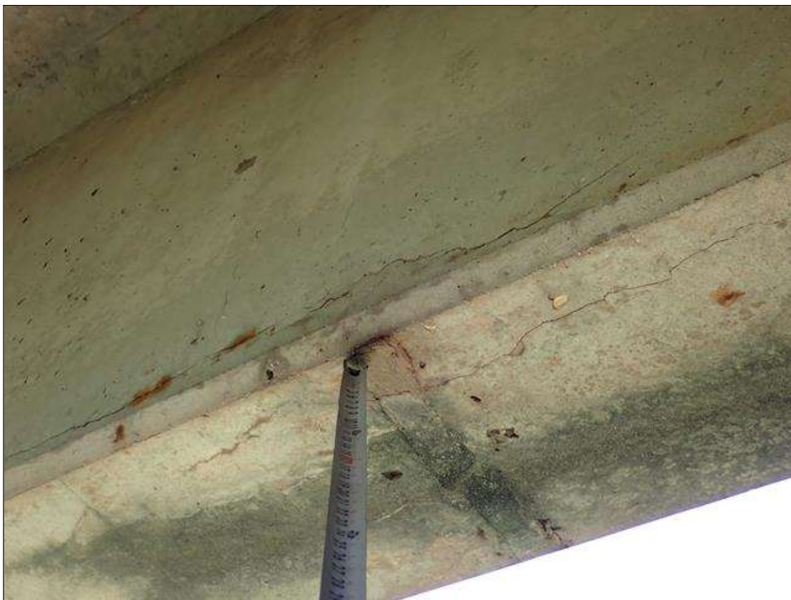
Span 2 Beam 4: (PAR) near bent 1, delamination (4 foot x 8 inch) and cracks (up to 1/16) with rust stains
