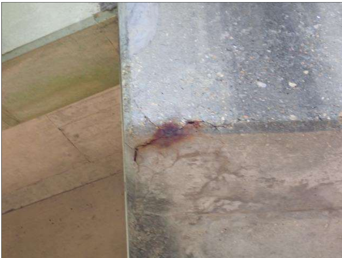
Bent 4 Cap 1: (PAR) west face at bottom corner, map cracks (up to 1/32 inch) with rust stains
