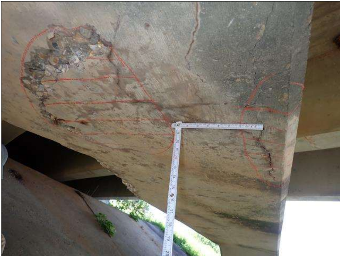
Bent 1 Cap 1: underside of cap near column 2, (2) spall/delamination (2 foot x 16 inch x 1/2 inch deep) with cracks (up to 1/16 inch)
