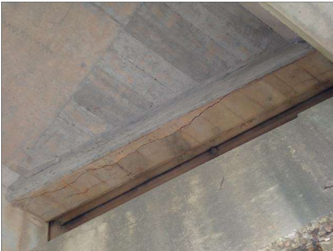
Span 3 Beam 2: at bents 2 and 3, bay 2 end diaphragms, spalls/delaminations (up to full length x full height) and cracks (up to 1/8 inch)
