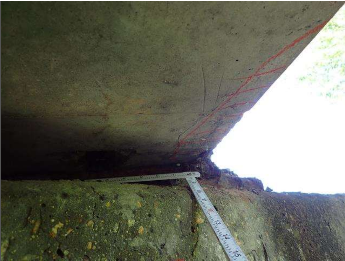
Span 5 Beam 1: at bent 4, underside, (2) spalls/delaminations (1 foot x 3 inch x 1/2 inch deep) with exposed rusted rebar
