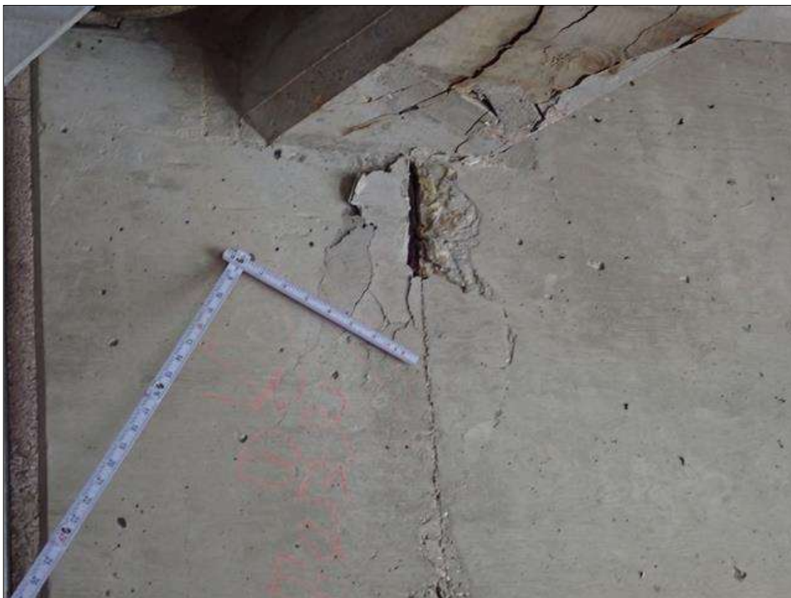
Span 2 Beam 2: East face at near end, delamination/spall [10 inch x 15 inch x up to 1/2 inch deep] with exposed rusted rebar
