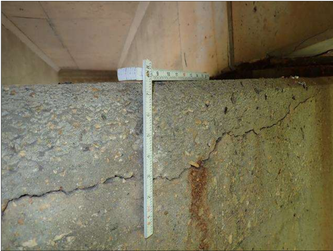
Bent 2 Cap 1: (PAR) (2)- UP TO 10 FOOT X 1/16 INCH HORIZONTAL CRACKS WITH RUST STAINS, SOUTH FACE, UNDER BAYS 2 AND 3.
