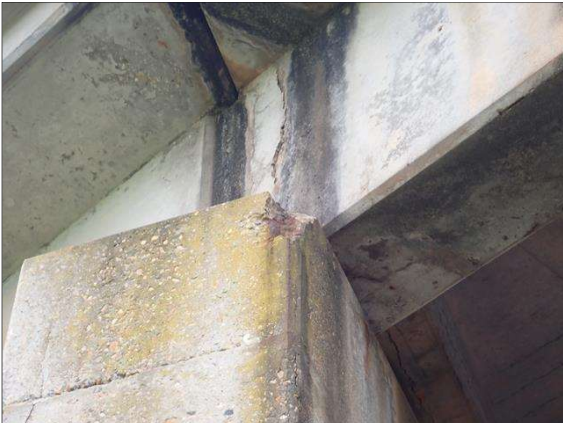
Bent 2 Cap 1: 9 INCH X 12 INCH X 2 INCH DEEP SPALL WITH EXPOSED REINFORCING ON NORTHEAST CORNER, NO LOSS NOTED ON REBAR
