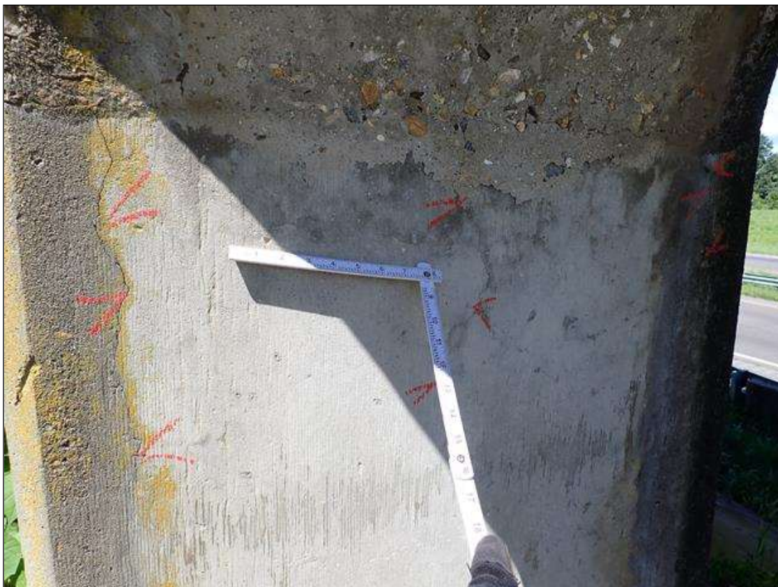
Bent 1 Pile 2: UP TO 4 FOOT X UP TO 1/32 INCH VERTICAL CRACKS, AT RANDOM THROUGHOUT.
