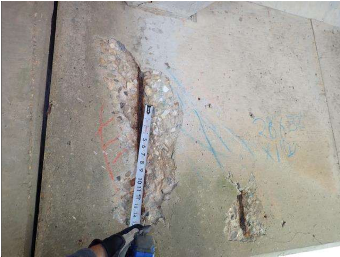
Span 3 Beam 4: (PAR) at bent 3, west face, (2) spalls/delaminations (1 foot x 30 inch x 1 inch deep) with exposed rusted rebar (approximately 25 percent loss) and cracks (up to 1/32 inch)
