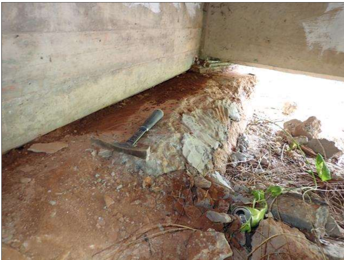
End Bent 2 Cap 1: (PAR) top of South face at bay 3, spall/delamination [10 foot x full height x full width x up to 3 inch deep] with exposed rusted rebar (approximately 25 percent loss) and cracks (up to 1/18 inch)
