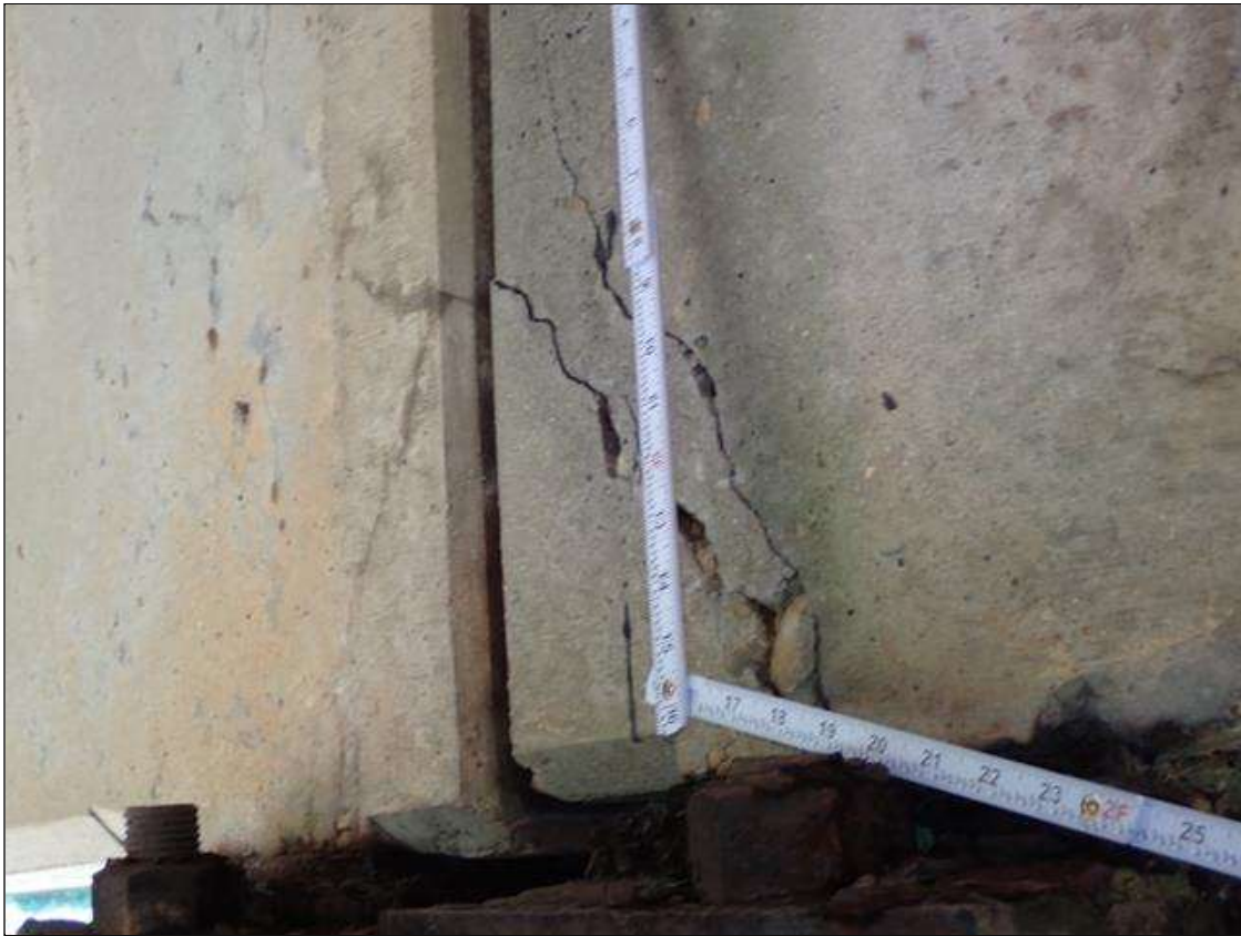
Span 1 Beam 4: (PAR) at bent 1, west and east faces and underside, multiple spalls/delaminations (up to 8 inch x 12 inch x 1/2 inch deep) with exposed rusted rebar (approximately 25 percent loss) and cracks (up to 1/8 inch)
