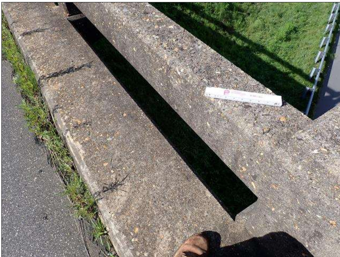
Span 2 Left Bridge Rail: (NOT FOUND 2023) LEFT RAIL HAS SCATTERED MAP CRACKING UP TO 1/64 INCH
