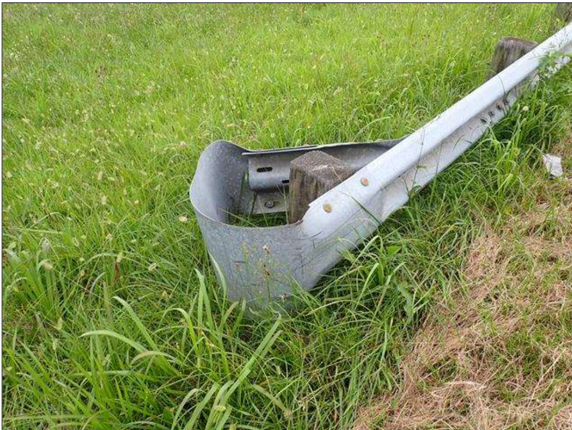
northeast guardrail termination
