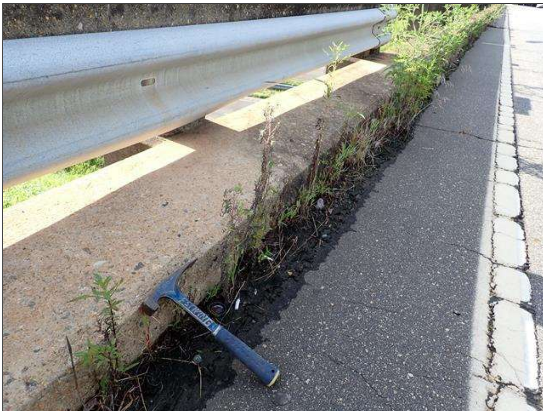
along curblines, debris accumulation (up to 1 foot x full length) with vegetation growth; partially obstructing drainage
