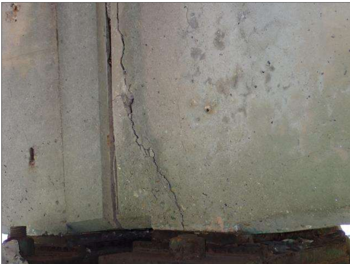
Span 2 Beam 2: West and east faces over bent 2, spalls/delaminations [up to 30 inch high x 7 inch wide x 3 inch deep] with cracks (up to 1/8 inch)
