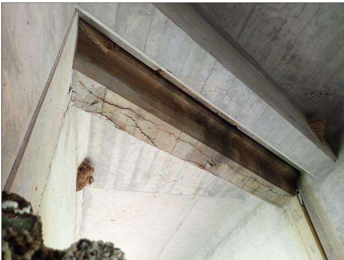
Span 2 Beam 2: at bents 1 and 2, bay 2 end diaphragm, delaminations (up to full length x full width) with cracks (up to 1/8 inch)
