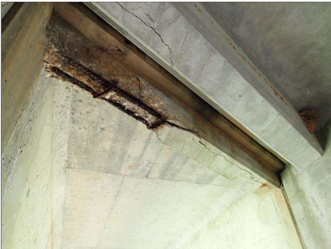
Span 2 Beam 1: (PAR) at bents 1 and 2, bay 1 end diaphragm, spalls/delaminations (up to full length x up to full height x 3 inch deep) with exposed rusted rebar (approximately 25 percent loss) and cracks (up to 1/8 inch) with rust stains
