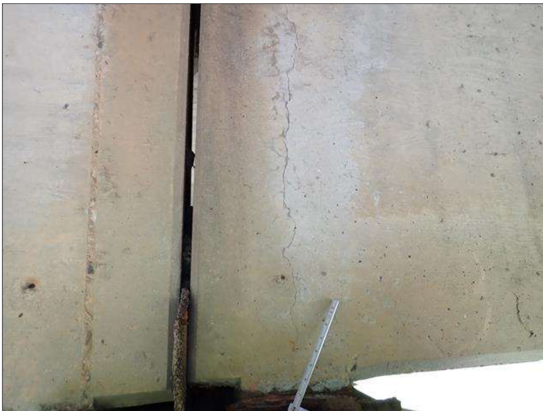
Span 3 Beam 2: TRANSVERSE AND WRAPAROUND CRACKS UP TO 1/32 INCH, AT RANDOM THROUGHOUT.
