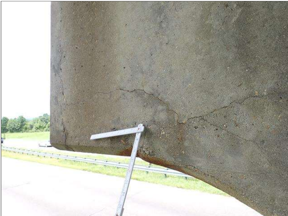
Bent 2 Cap 1: (PAR) southwest corner, spall/delamination (18 inch x 6 inch x 1 inch deep) with exposed rusted rebar and adjacent map cracks (up to 1/32 inch) with rust stains
