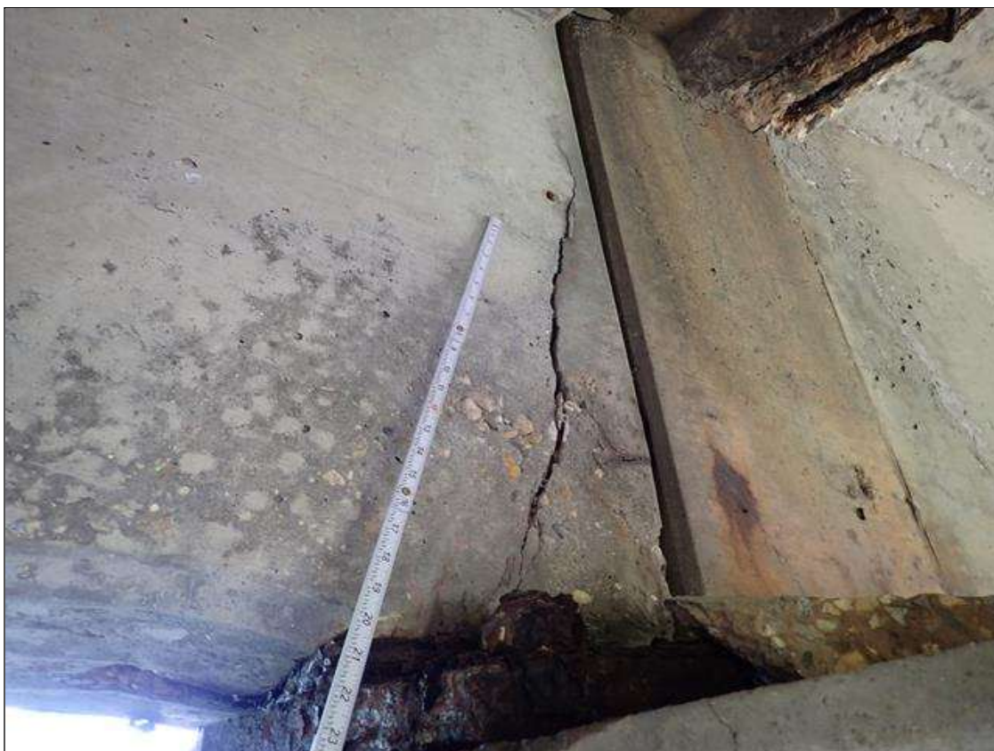
Span 1 Beam 1: at bent 1, east face, delamination (26 inch x 6 inch) with cracks (up to 1/2 inch)
