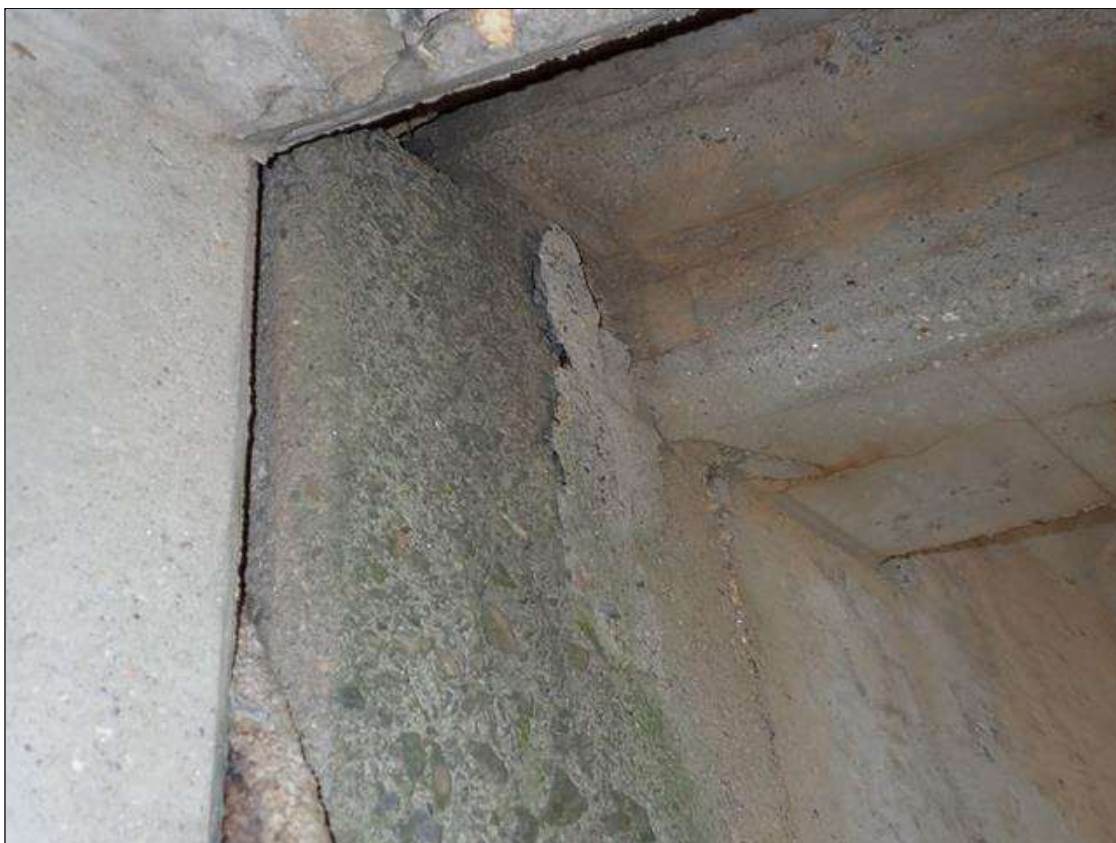
Span 3 Beam 1: at bent 2, east face at top, delamination (12 inch x 4 inch)
