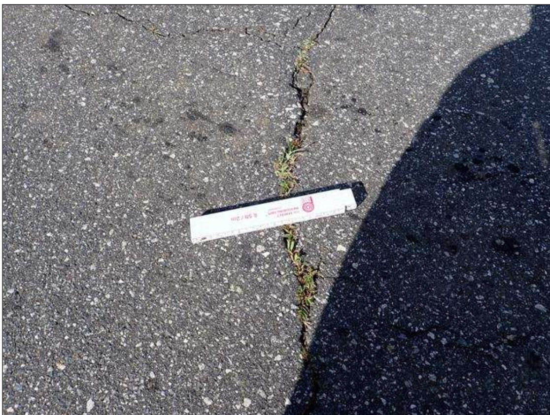
Span 5 Wearing Surface: 30 FOOT X UP TO 1/4 INCH TRANSVERSE CRACK OVER END BENT 2.
