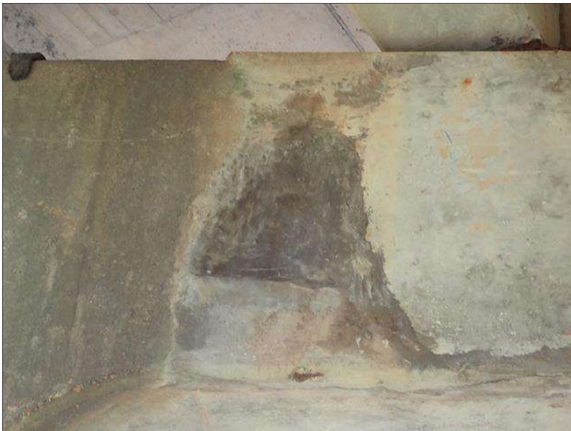
Bent 4 Cap 1: 2 FOOT X 2 FOOT UNSOUND PATCH, NORTH FACE, UNDER BAY 3.
