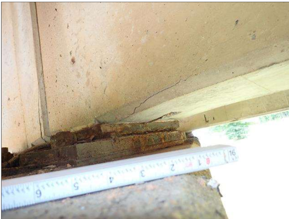
Span 2 Beam 3: at bent 2, underside, (2) spalls/delaminations (up to 1 foot x 6 inch x 1/2 inch deep) with exposed rusted rebar
