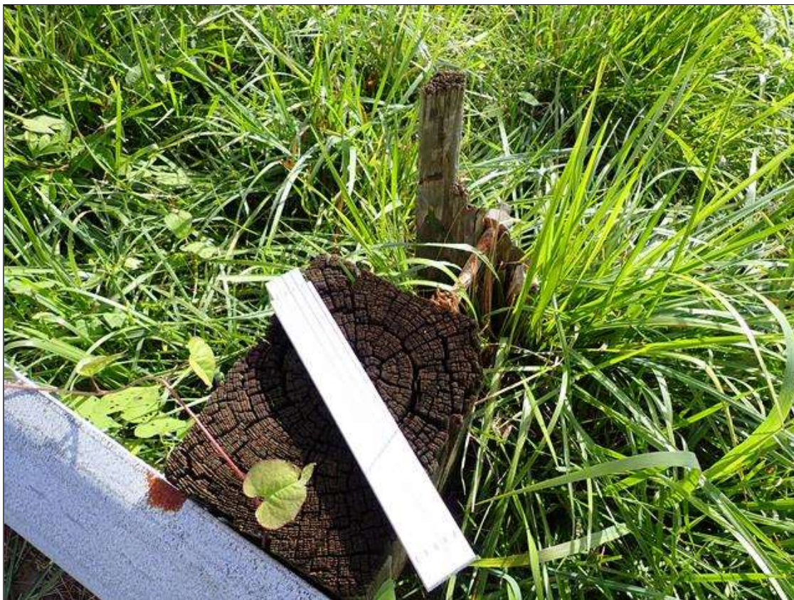
(PAR) northeast guardrail, 3rd and 12th timber posts from end bent 2, decay/section loss (up to full width x full height x full depth)
