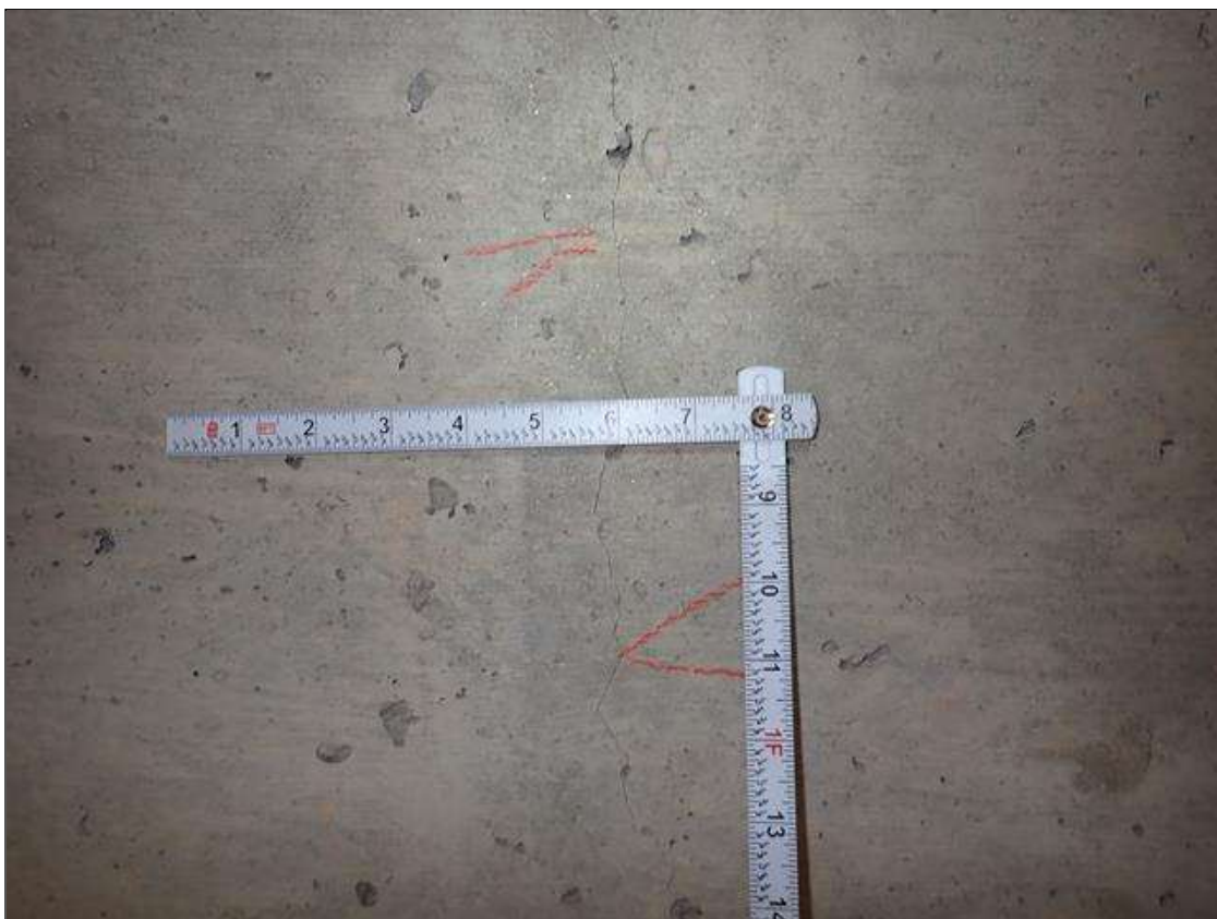
Span 1 Beam 4: along the length of the beam, vertical cracks (up to 1/64 inch x full height) at random
