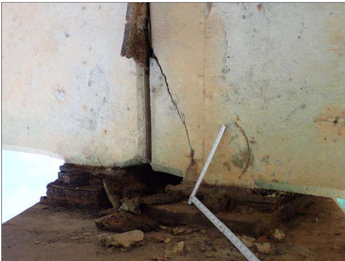
Span 5 Beam 3: East face over bent 4, delamination [16 inch x 8 inch] with cracks (up to 1/8 inch)
