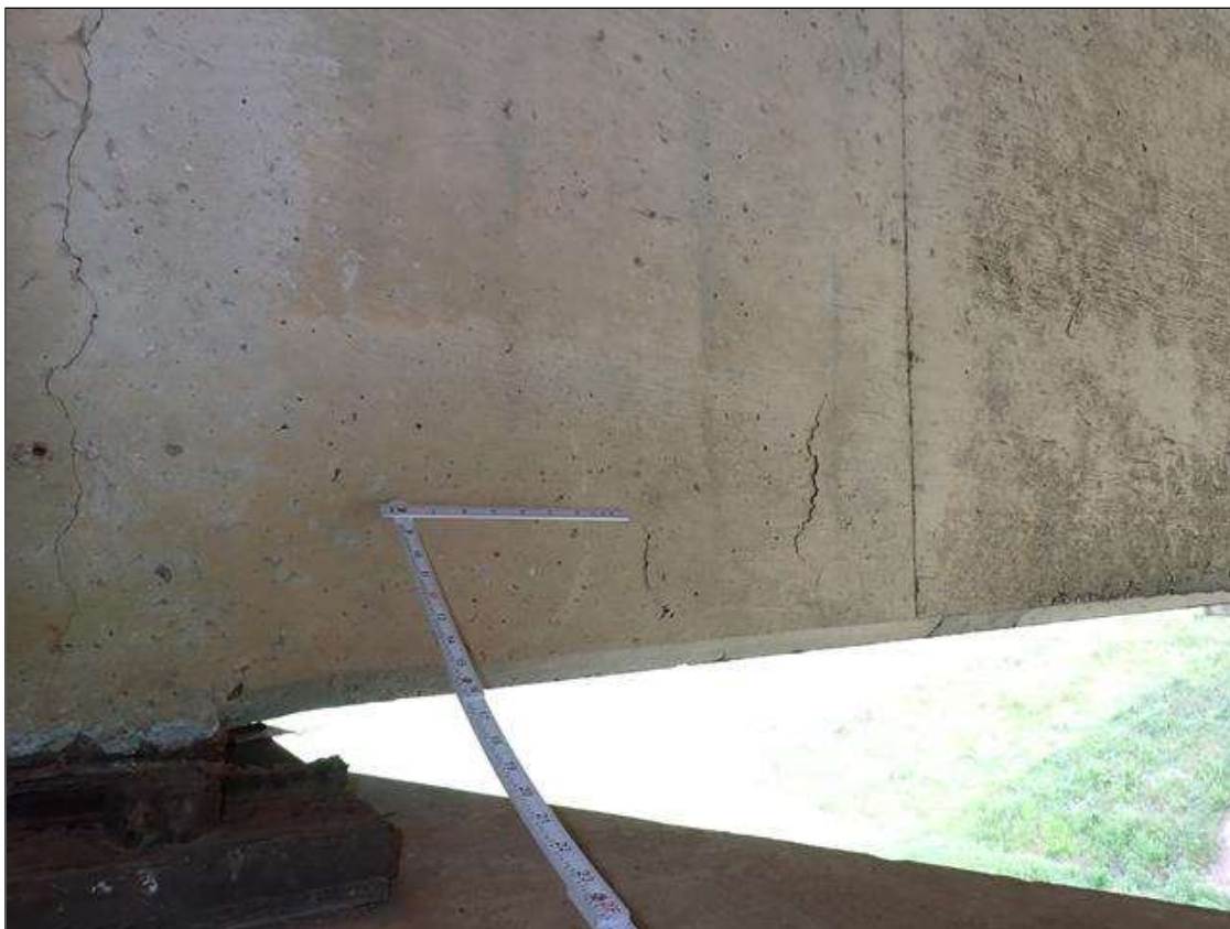
Span 3 Beam 2: near bent 3, west face, (3) delaminations (8 inch diameter) with cracks (up to 1/32 inch)
