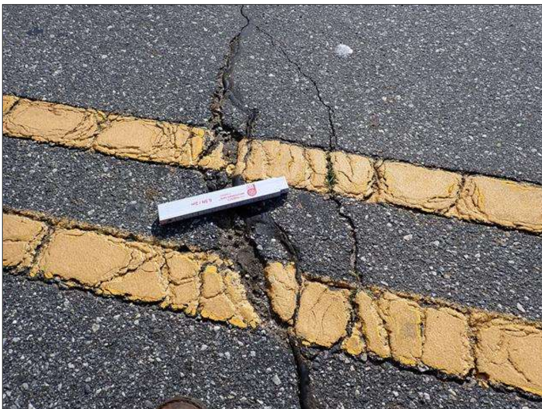
Span 4 Wearing Surface: over bent 4, partially sealed transverse crack (1/8 inch x full width) with edge spalling (up to 2 foot x 2 inch x 1/2 inch deep) with vegetation growth
