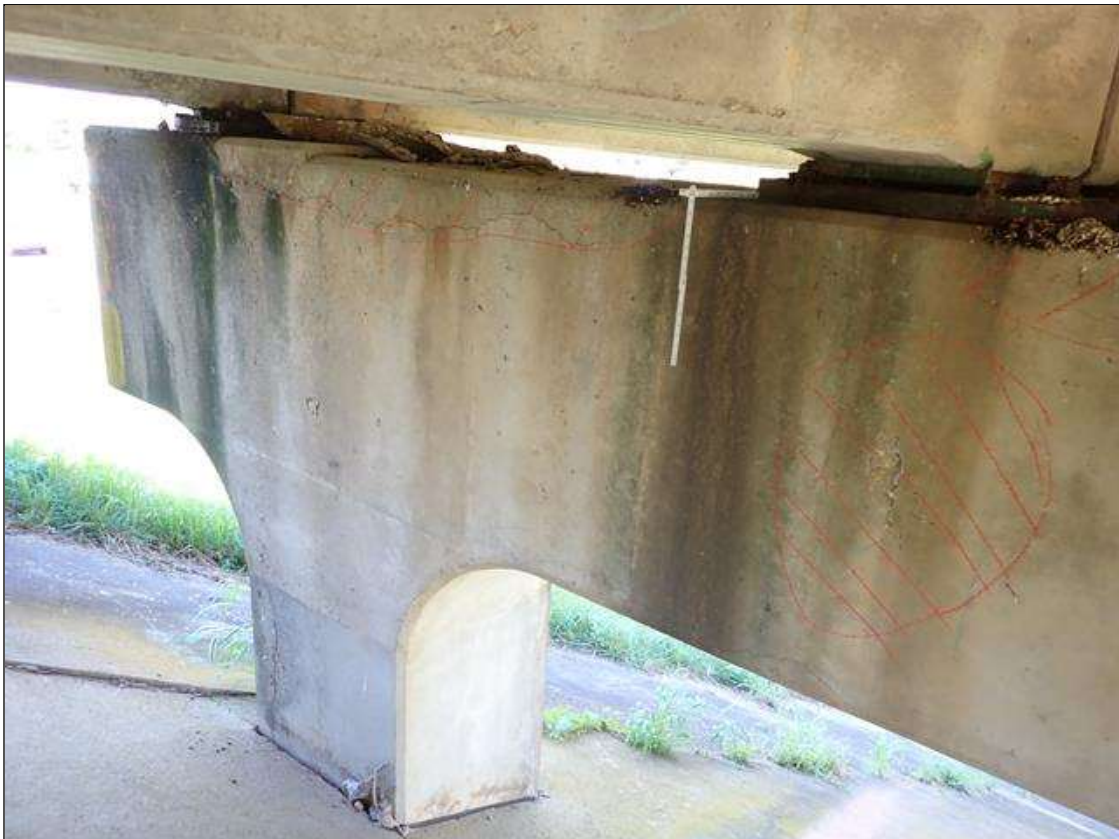
Bent 1 Cap 1: (PAR) along north and south faces, multiple spalls/delaminations (up to 16 foot x full height x 2.5 inch deep) with exposed rusted rebar (approximately 25 percent loss) and cracks (1/8 inch) at random
