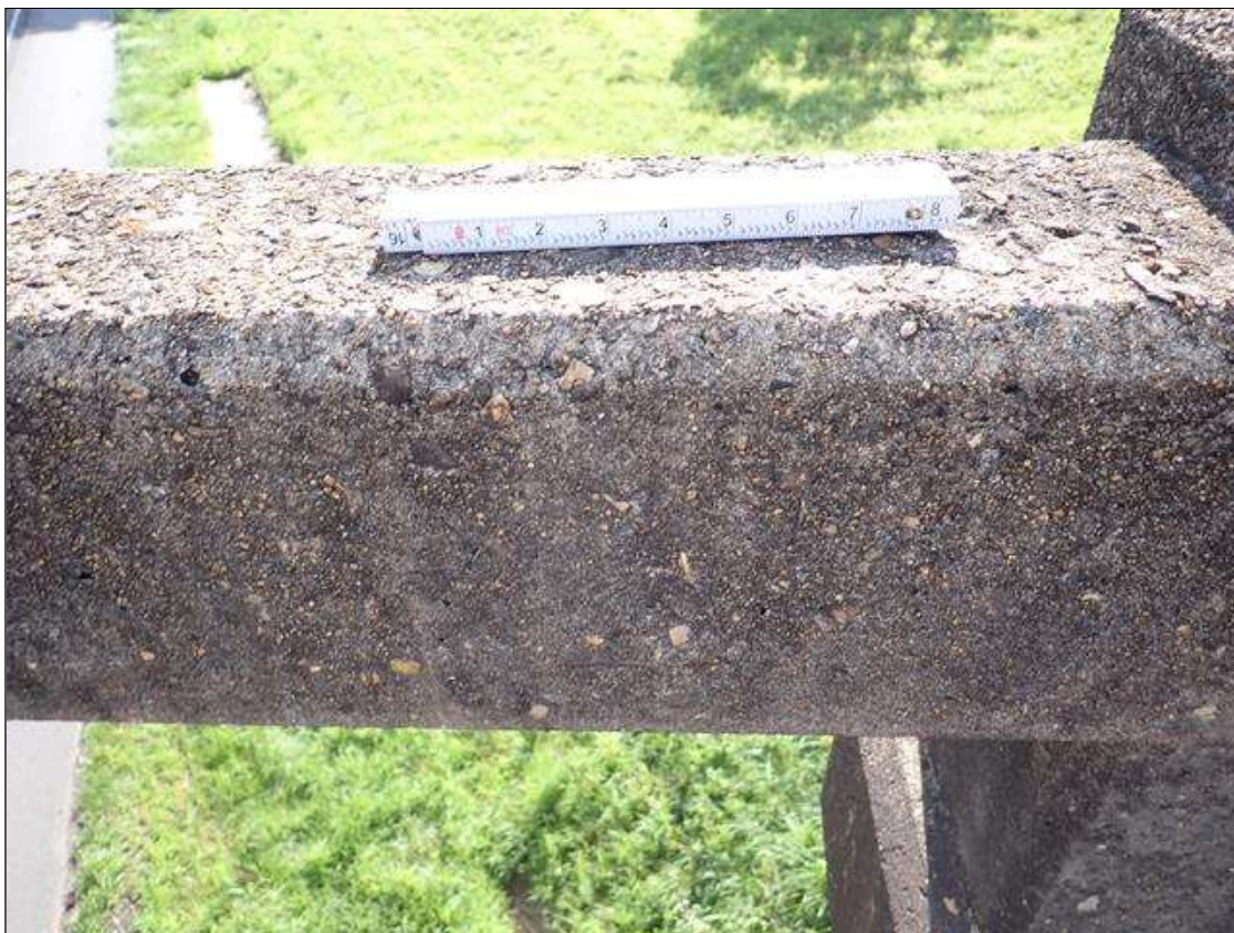
Span 2 Right Bridge Rail: (NOT FOUND 2023) RIGHT RAIL HAS SCATTERED MAP CRACKING UP TO 1/64 INCH
