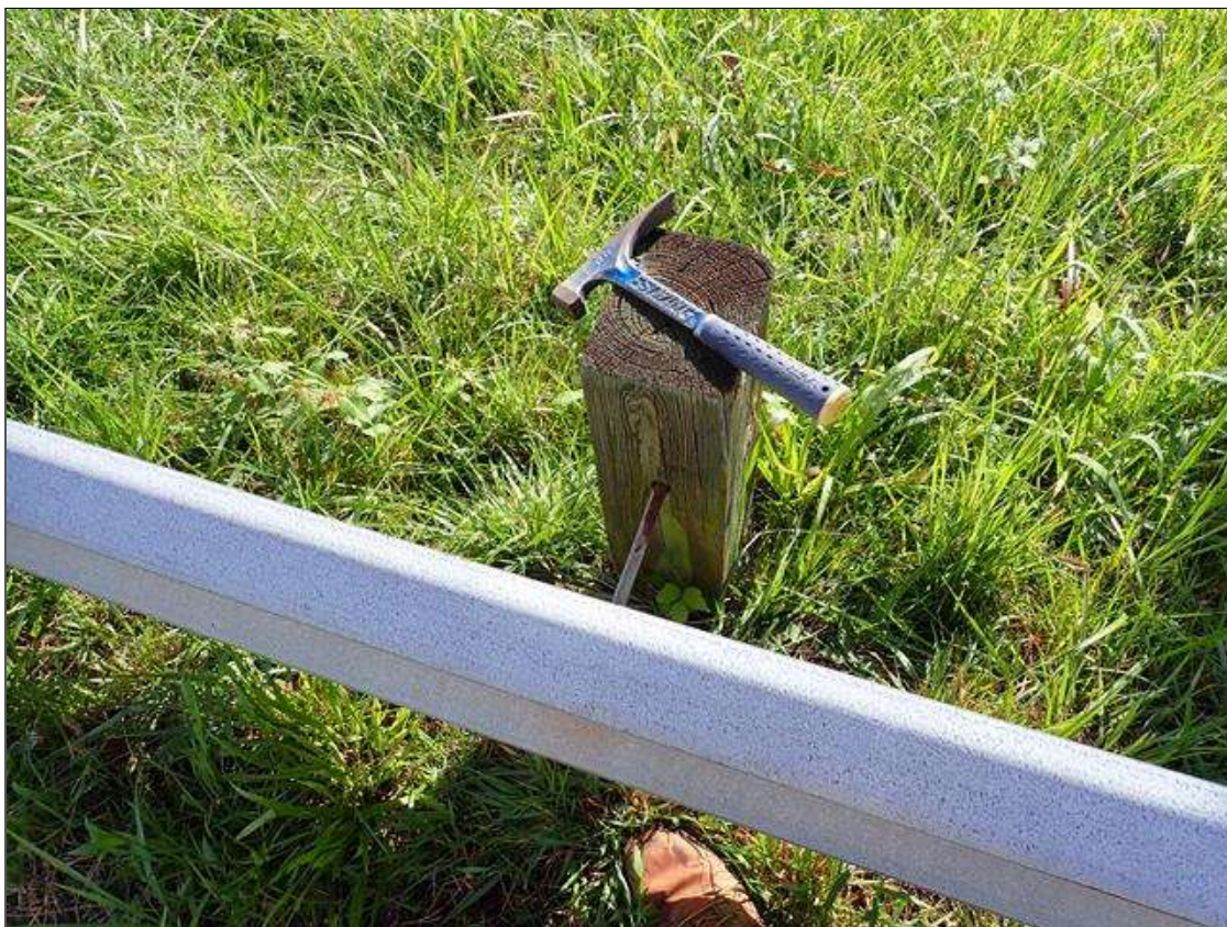
(PAR) southeast guardrail, 9th timber spacer from end bent 1, missing
