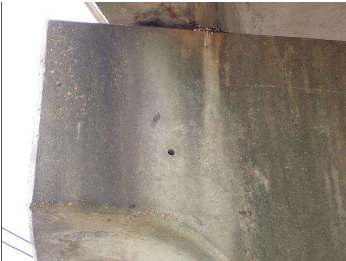
Bent 4 Cap 1: (not found 2023) North face under beam 4, delamination/spall [up to 15 inch x 17 inch x 1/4 inch deep]
