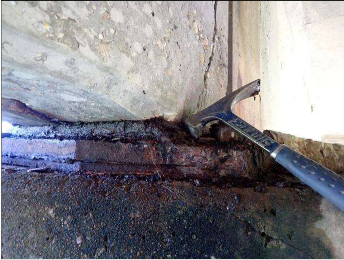
Span 1 Far Bearing 1: corrosion with section loss [up to 1/16 inch loss]
