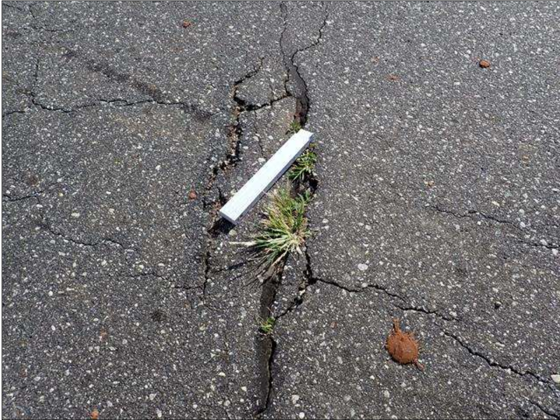
Span 3 Wearing Surface: over bent 3, partially sealed transverse crack (1/8 inch x full width) with edge spalling (up to 2 foot x 2 inch x 1/2 inch deep) with vegetation growth
