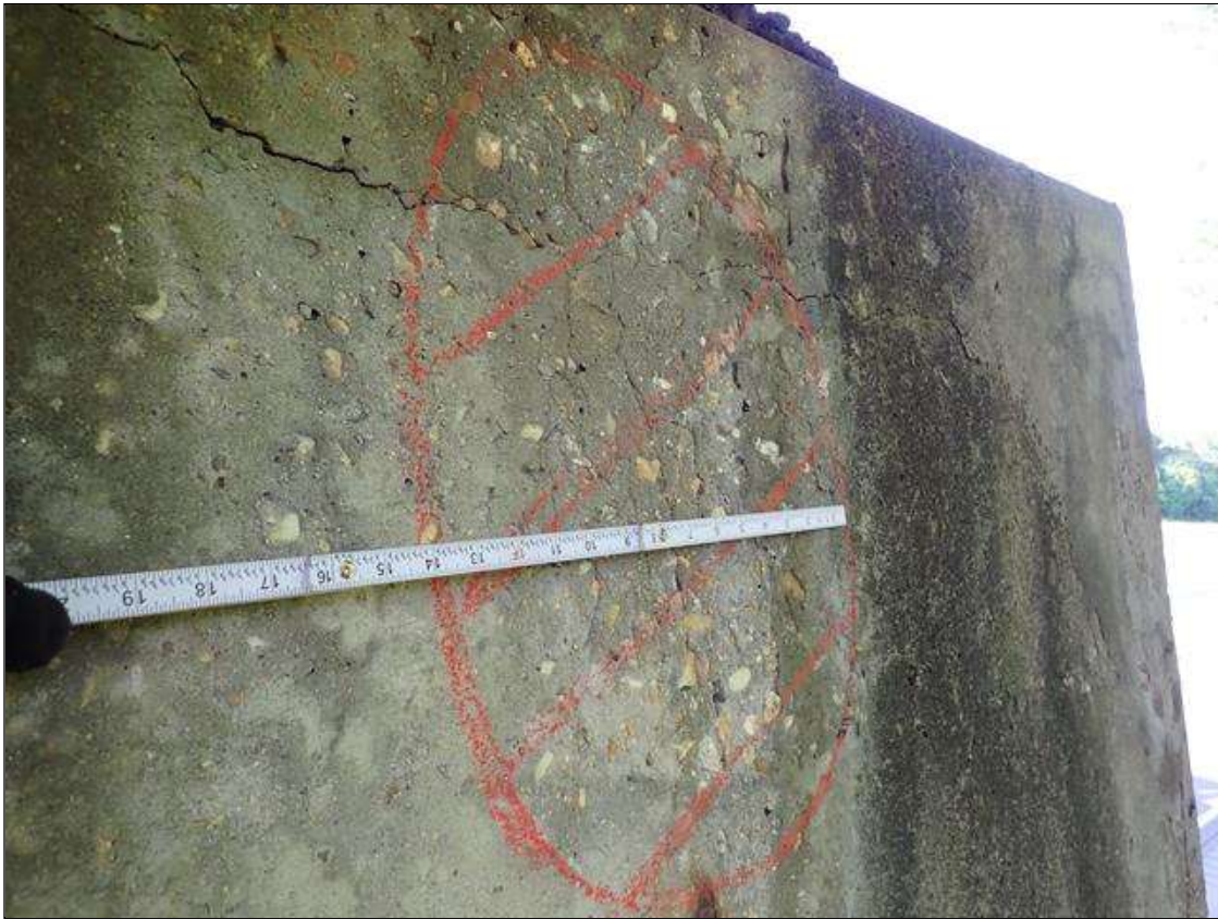
Bent 4 Cap 1: North face of cap under beam 1, delamination [14 inch x 18 inch]
