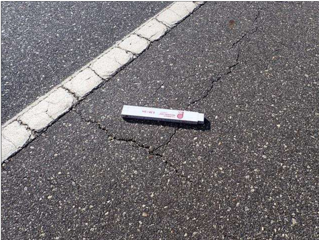
Span 4 Wearing Surface: WEARING SURFACE HAS SCATTERED TRANSVERSE AND LONGITUDINAL CRACKS UP TO 1/8 INCH
