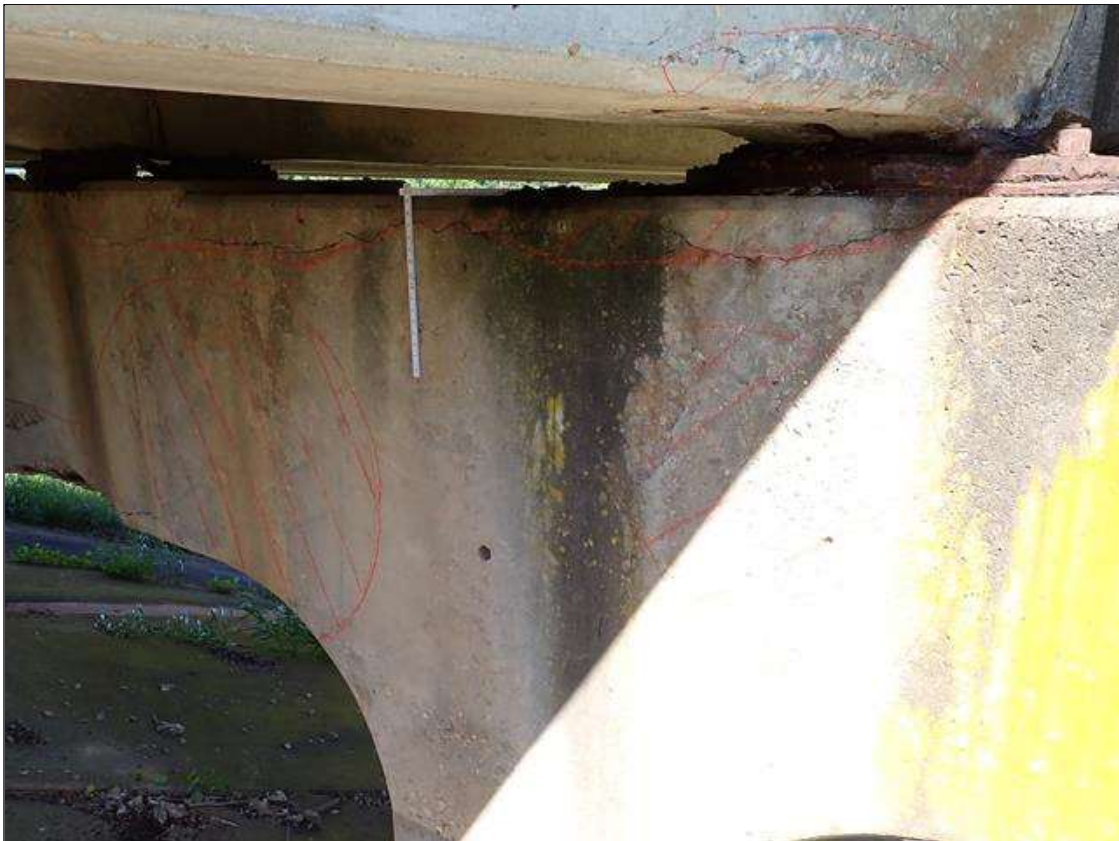
Bent 1 Cap 1: (PAR) along north and south faces, multiple spalls/delaminations (up to 16 foot x full height x 2.5 inch deep) with exposed rusted rebar (approximately 25 percent loss) and cracks (1/8 inch) at random
