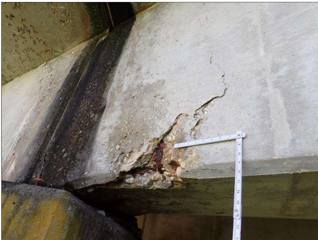
Span 1 Beam 1: (PAR) at bent 1, west face and underside, (2) spalls/delamination (up to 2.5 foot x 2 foot x 2 inch deep) with exposed rusted rebar (approximately 25 percent loss)
