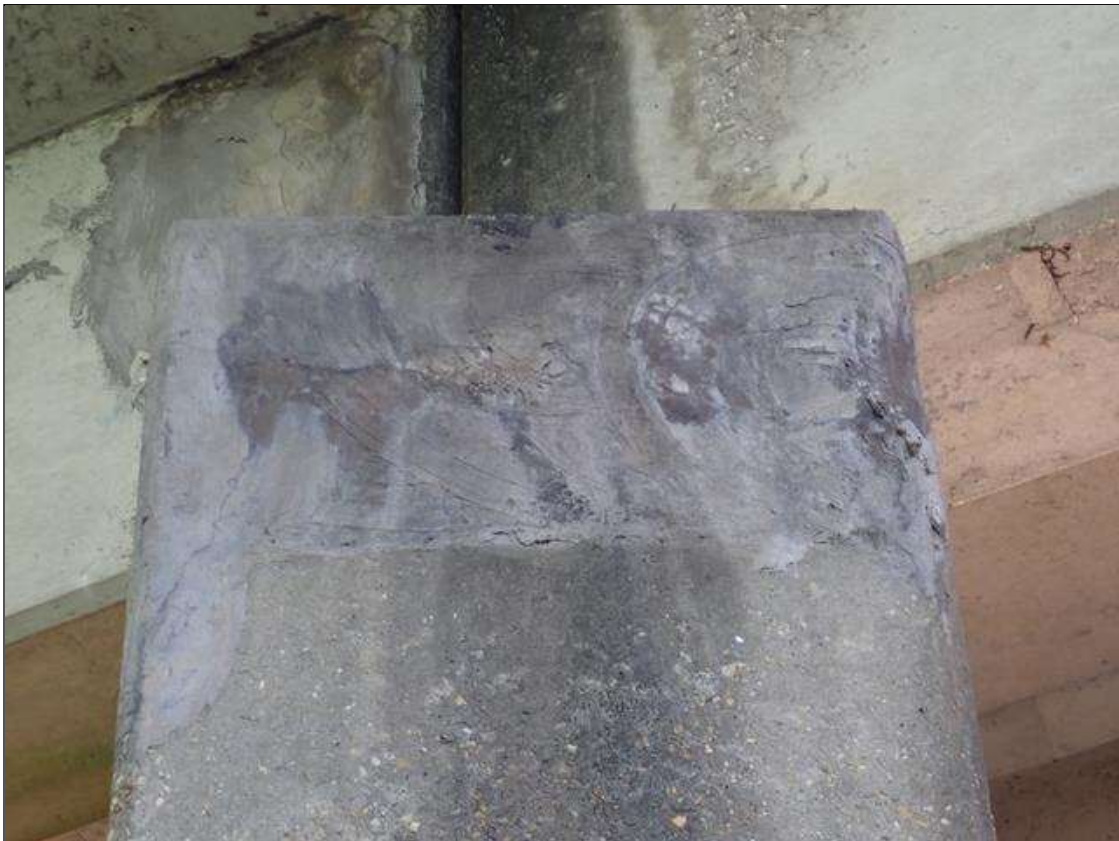
Bent 4 Cap 1: WEST FACE HAS A PATCHED AREA (3 FOOT X 2 FOOT) WITH HAIRLINE MAP CRACKING. PATCH APPEARS TO BE SOUND.
