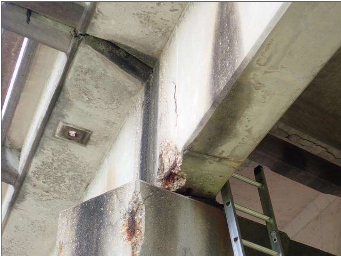
Span 2 Beam 1: (PAR) at bent 2, west face and underside, multiple spalls/delaminations (2 foot x 32 inch x 2.5 inch deep) with exposed rusted rebar (approximately 25 percent loss) and cracks (up to 1/8 inch)
