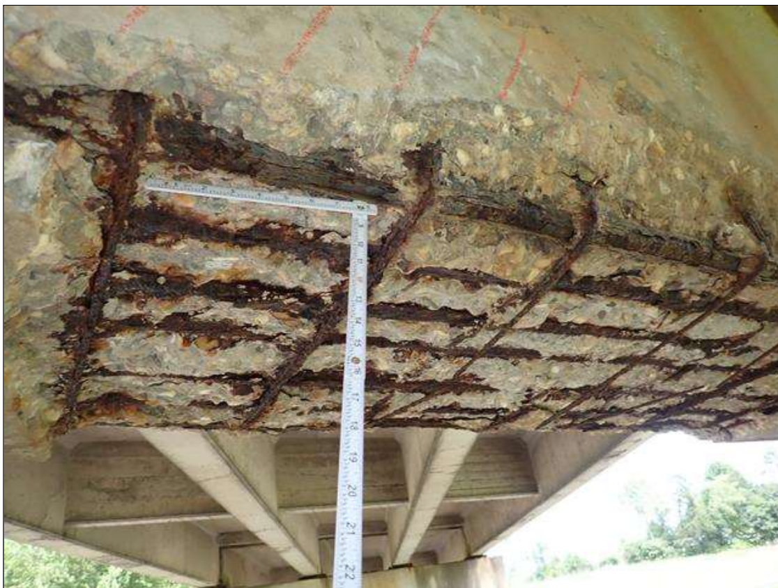
Bent 2 Cap 1: (PAR) underside of cap between columns, spall/delamination [14 foot long x full width x up to 4 inch deep] that extends onto south face [13 inch] with exposed rusted rebar and stirrups [rebars with approximately 25 percent loss; stirrups up to 100 percent loss]
