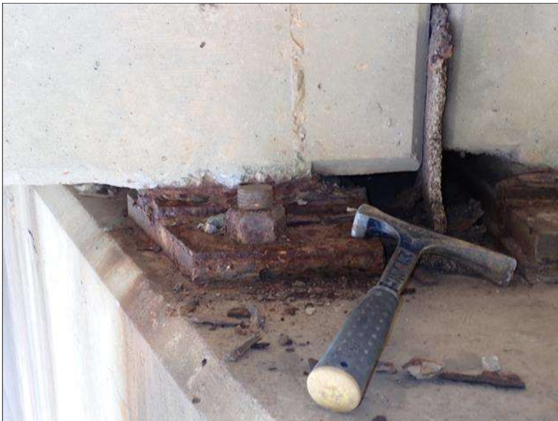
Span 4 Near Bearing 2: corrosion with section loss (up to 1/16 inch loss)
