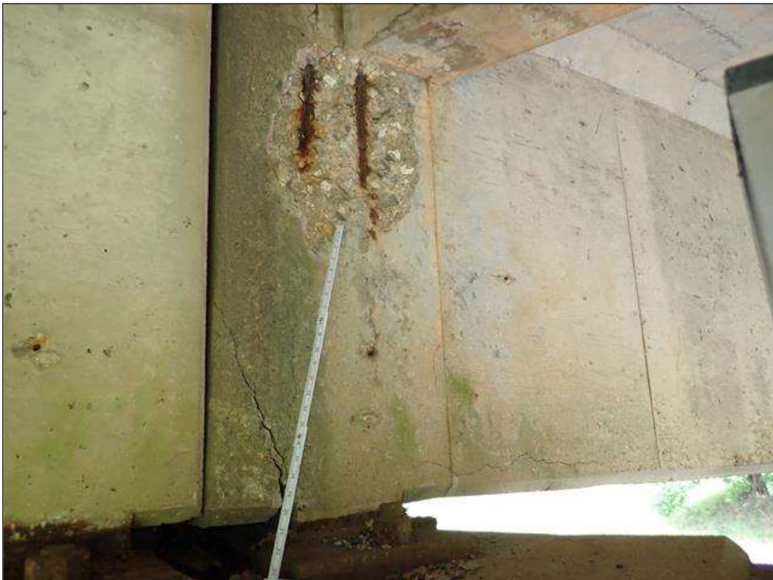
Span 3 Beam 3: (PAR) East face over bent 2, (3) spalls/delaminations [up to 17 inch long x 24 inch high x up to 2 inch deep] with exposed rusted rebar [approximately 25 percent loss] and cracks [up to 1/16 inch]
