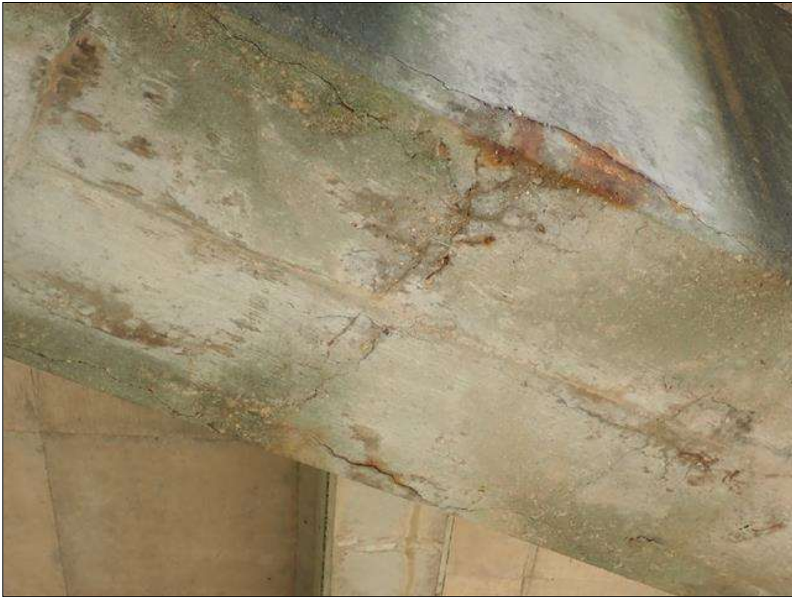
Bent 4 Cap 1: (PAR) underside of cap between columns 1 and 2, longitudinal cracks (up to 1/16 inch x 4 foot) some with rust stains and adjacent delaminations (up to 8 foot x full width)
