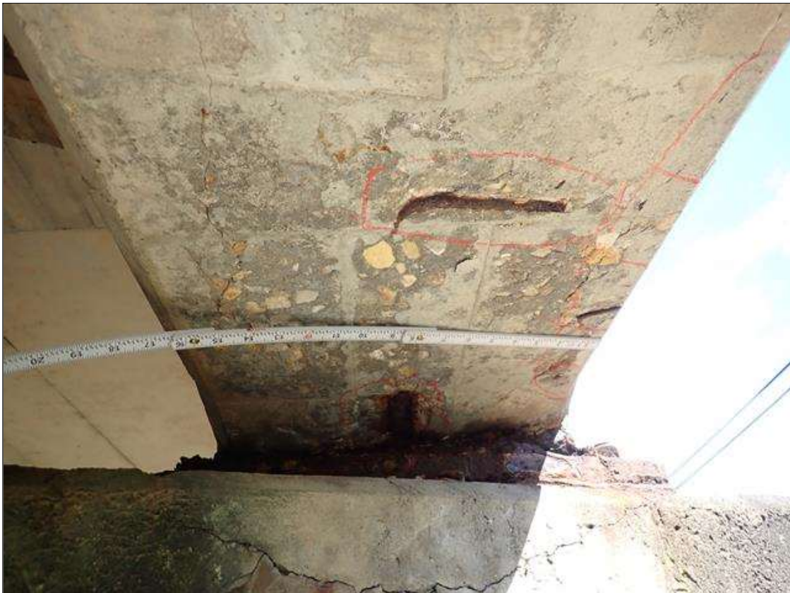
Span 1 Beam 4: (PAR) at bent 1, west and east faces and underside, multiple spalls/delaminations (up to 8 inch x 12 inch x 1/2 inch deep) with exposed rusted rebar (approximately 25 percent loss) and cracks (up to 1/8 inch)
