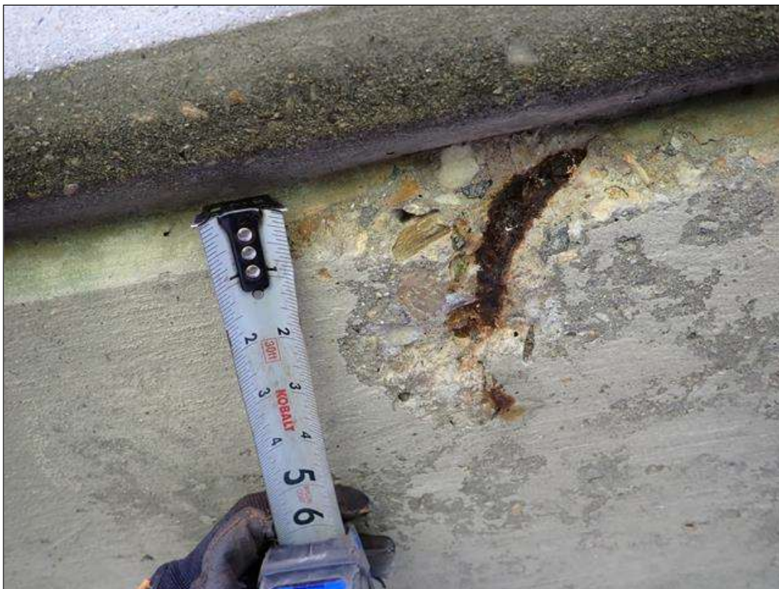
Span 1 Deck: (PAR) west overhang 10 foot from end bent 1, spall (5 inch x 5 inch x 1/2 inch deep) with exposed rusted rebar
