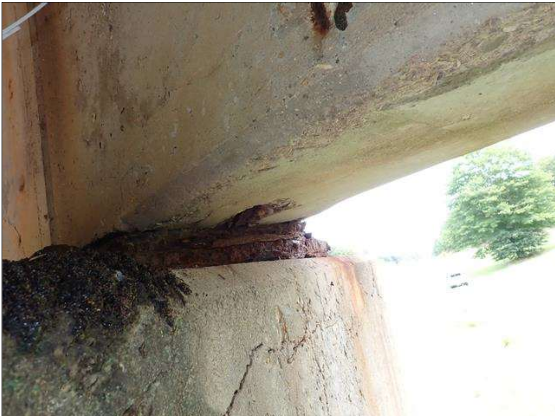
Span 2 Beam 4: (PAR) at bent 2, west and east faces and underside, multiple spalls/delaminations (up to 18 inch x 8 inch x 1 inch deep) with exposed rusted rebar (approximately 25 percent loss)
