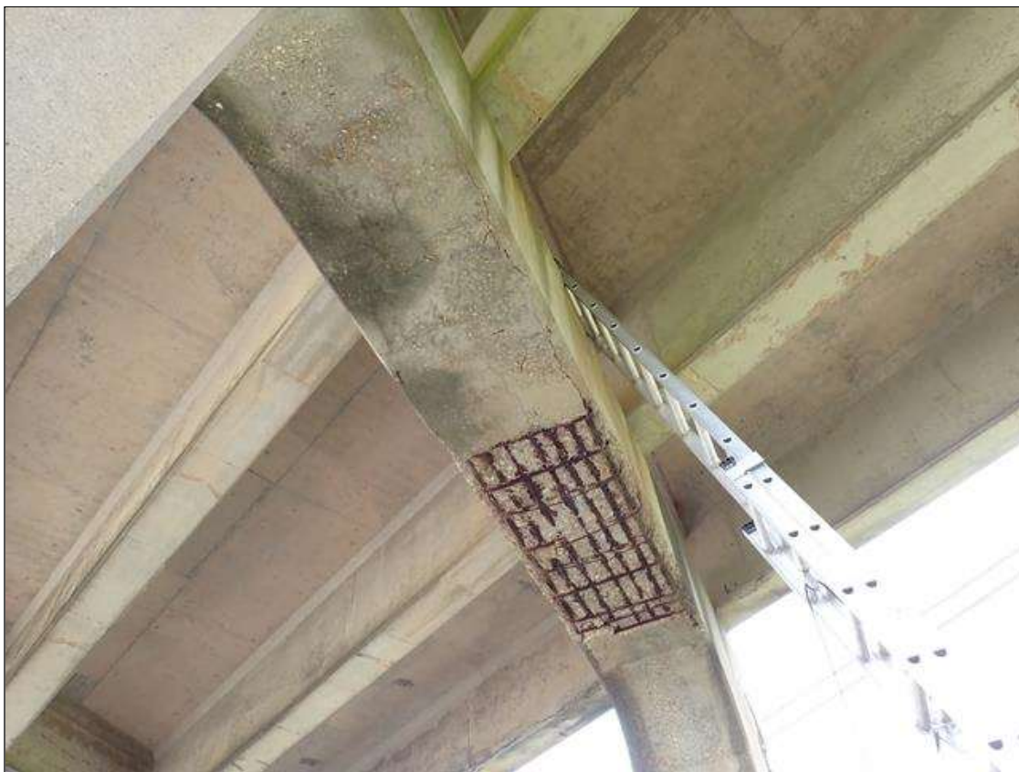
Bent 2 Cap 1: (PAR) underside of cap between columns, spall/delamination [14 foot long x full width x up to 4 inch deep] that extends onto south face [13 inch] with exposed rusted rebar and stirrups [rebars with approximately 25 percent loss; stirrups up to 100 percent loss]
