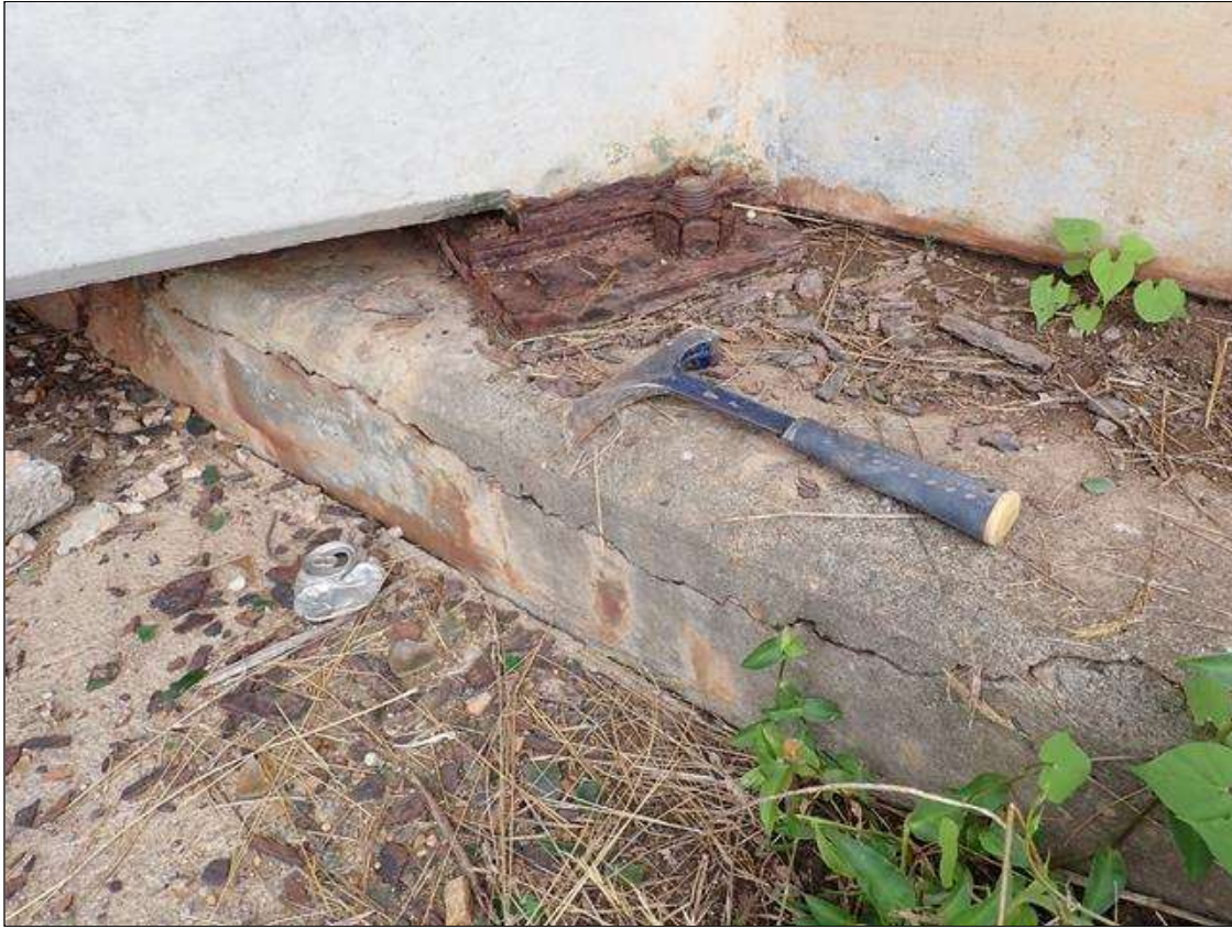
End Bent 2 Cap 1: (PAR) top of South face at bay 3, spall/delamination [10 foot x full height x full width x up to 3 inch deep] with exposed rusted rebar (approximately 25 percent loss) and cracks (up to 1/18 inch)
