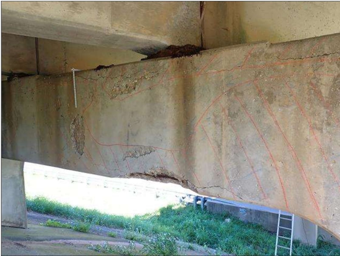
Bent 1 Cap 1: (PAR) along north and south faces, multiple spalls/delaminations (up to 16 foot x full height x 2.5 inch deep) with exposed rusted rebar (approximately 25 percent loss) and cracks (1/8 inch) at random
