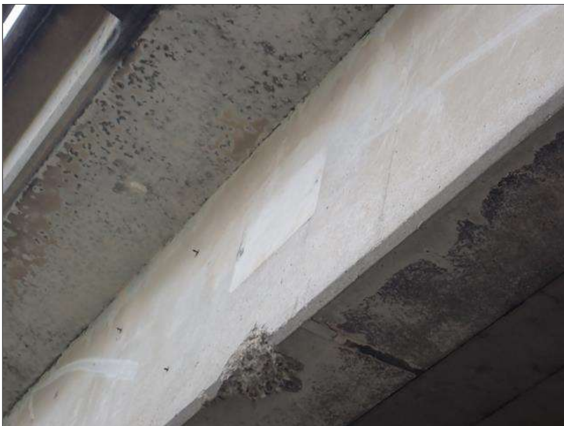
Span 4 Route Marker Sign: (PAR) route sign, missing
