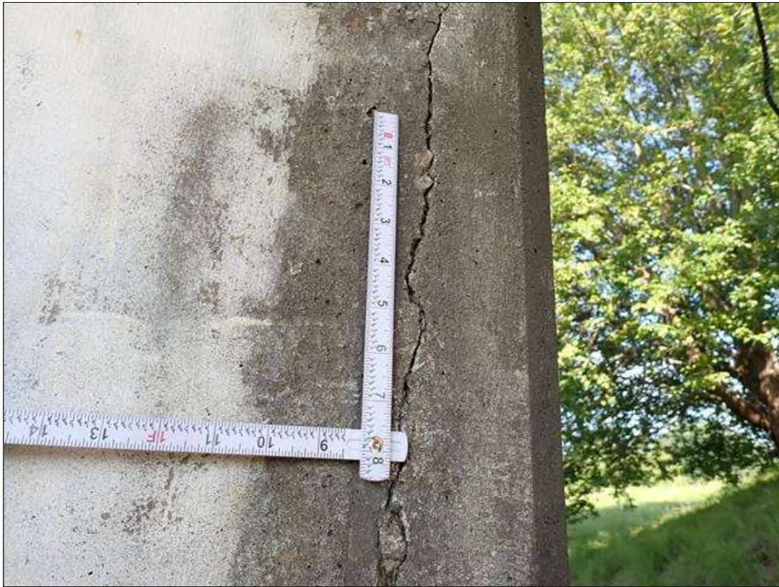
Bent 4 Pile 1: UP TO 10 FOOT X UP TO 1/16 INCH VERTICAL CRACKS, AT RANDOM THROUGHOUT.
