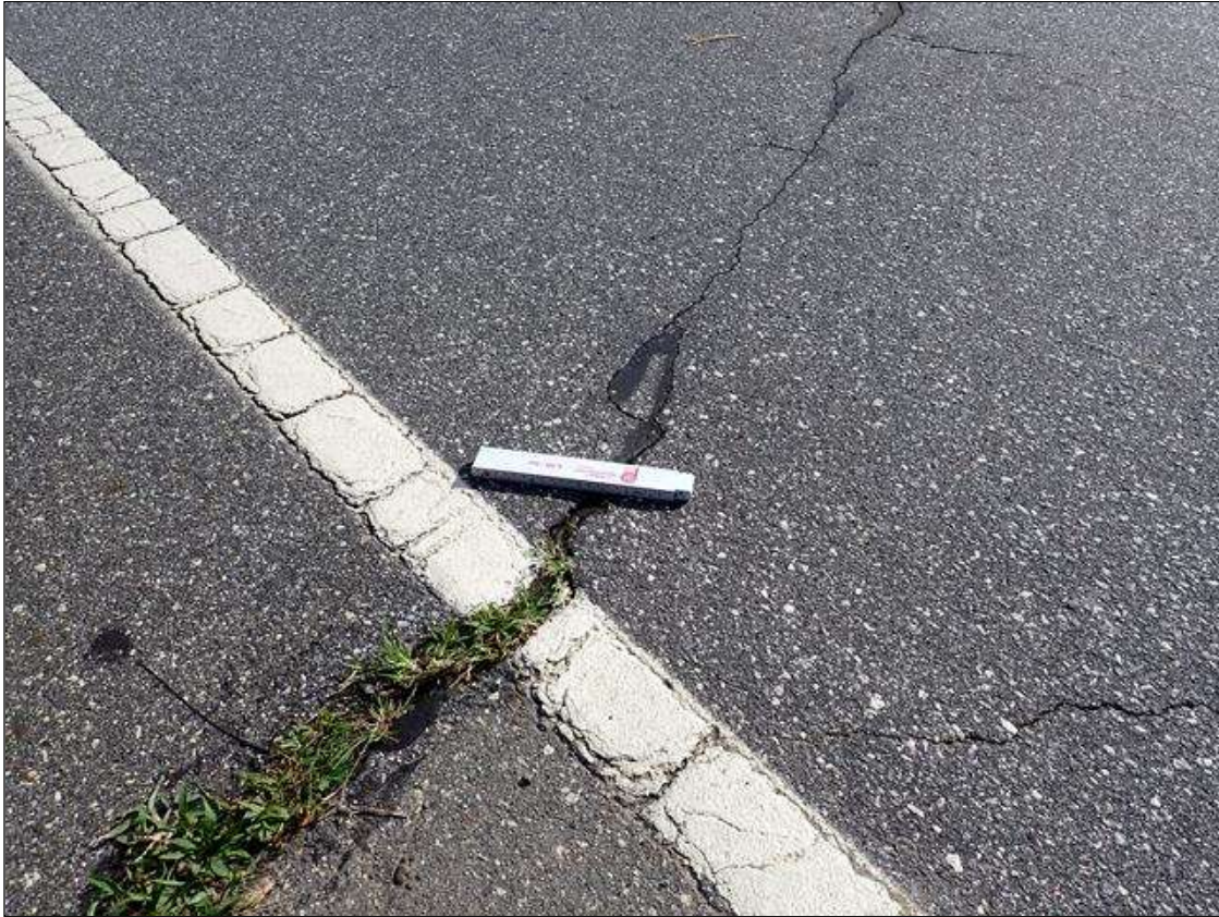
Span 4 Wearing Surface: over bent 4, partially sealed transverse crack (1/8 inch x full width) with edge spalling (up to 2 foot x 2 inch x 1/2 inch deep) with vegetation growth
