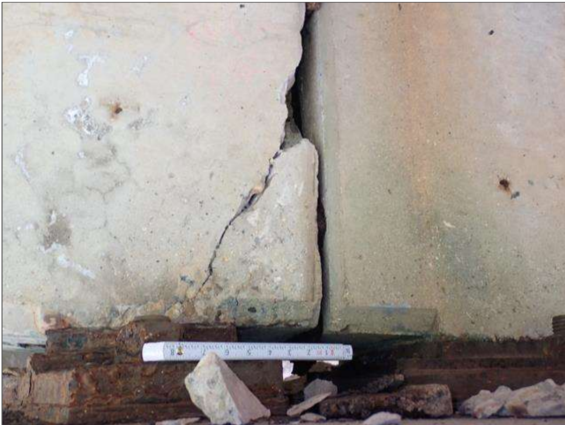
Span 2 Beam 2: West and east faces over bent 2, spalls/delaminations [up to 30 inch high x 7 inch wide x 3 inch deep] with cracks (up to 1/8 inch)
