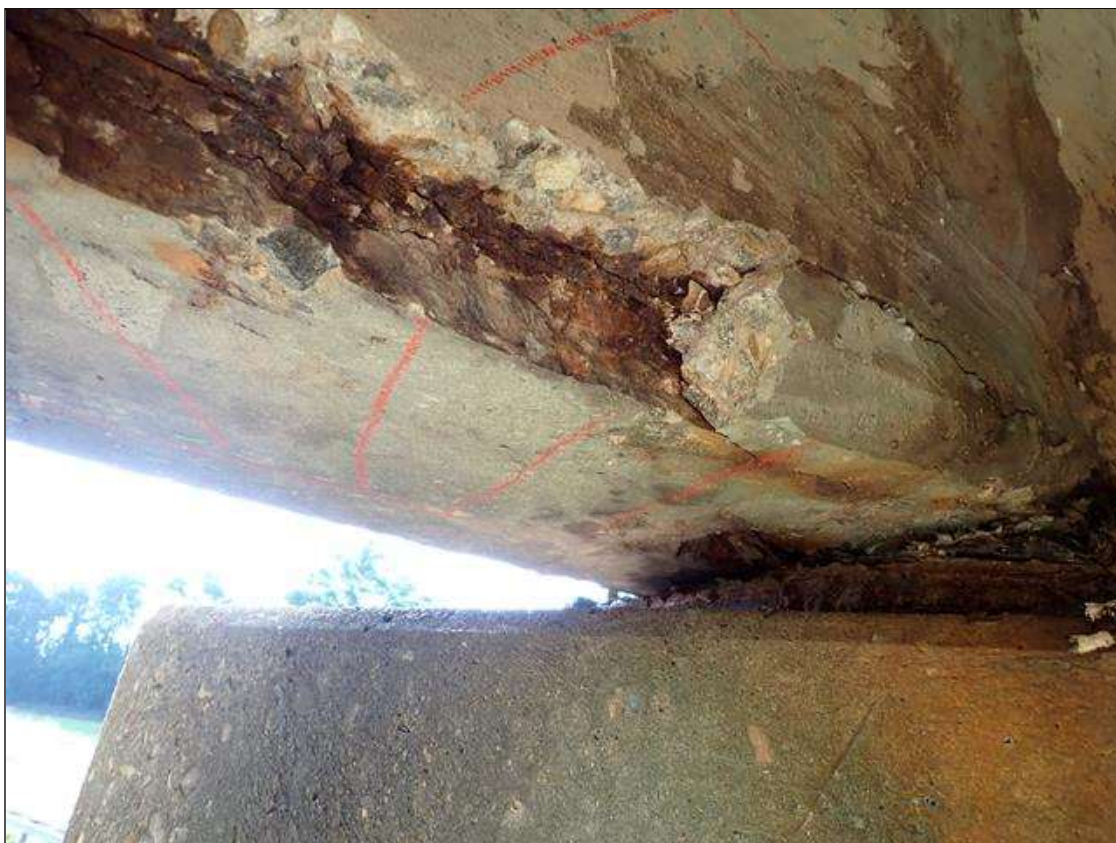
Span 5 Beam 4: (PAR) at bent 4, west face and underside, spall/delamination (6 foot x full width x up to 6 inch x 1.5 inch deep) with exposed rusted rebar (approximately 25 percent loss)
