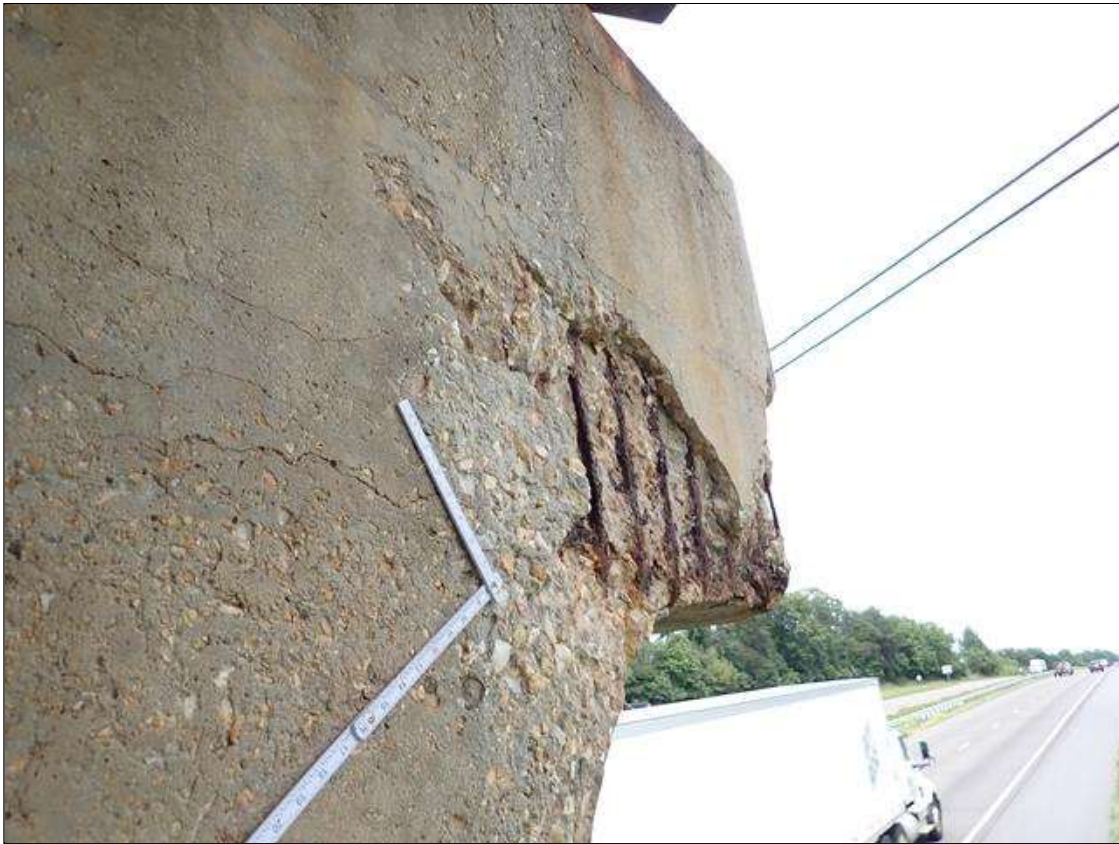
Bent 2 Cap 1: (PAR) South face at East end, spall/delamination [84 inch long x up to full height x up to 3 inch deep] with exposed rusted rebar and stirrups [rebar and stirrups with approximately 25 percent loss] and cracks [up to 1/8 inch]
