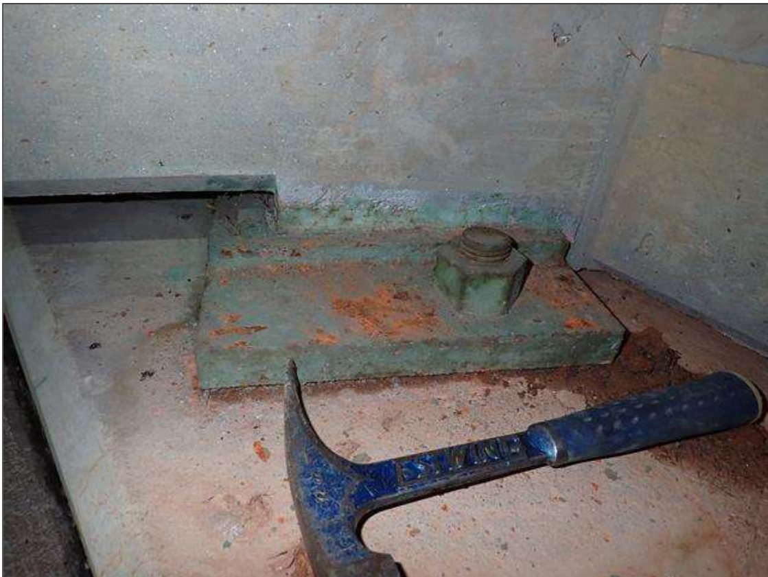
Span 1 Near Bearing 2: freckled rust
