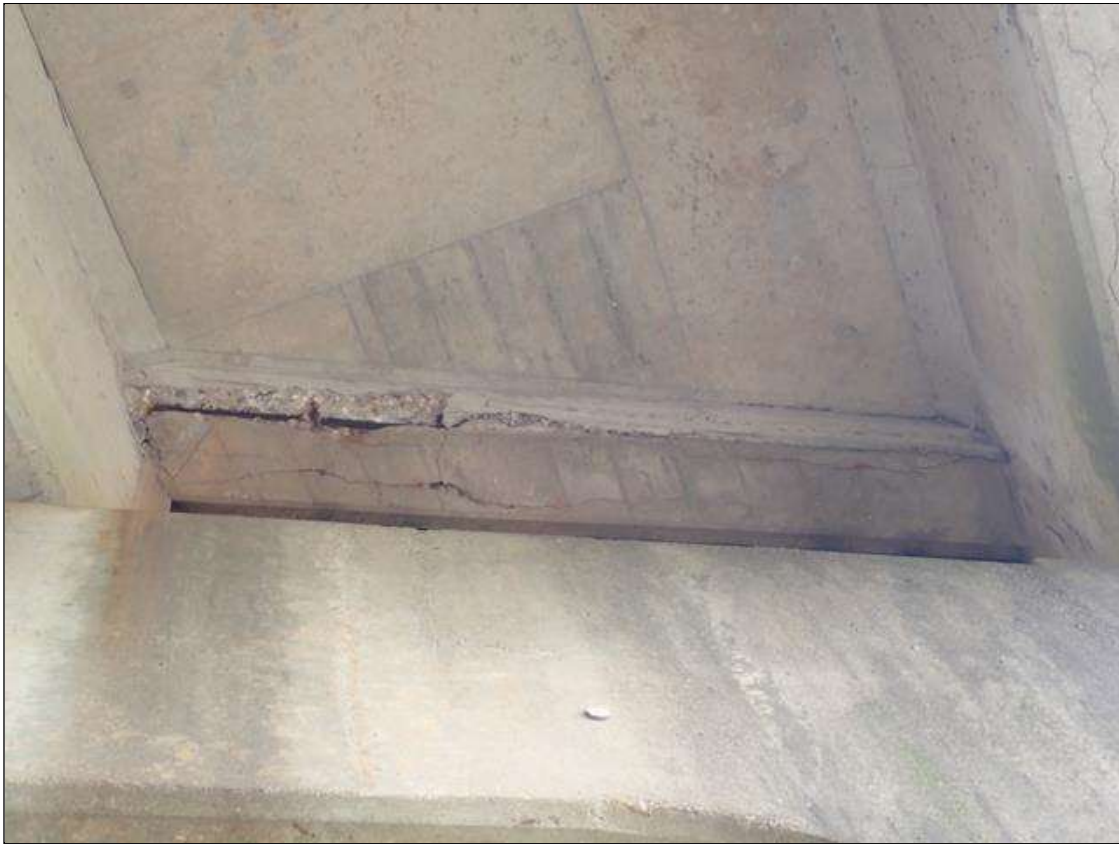
Span 4 Beam 1: (PAR) at bents 3 and 4, bay 1 end diaphragms, spalls/delaminations (up to full length x full height x up to 1.5 inch deep) with exposed rusted rebar (approximately 25 percent loss) and cracks (up to 1/8 inch) and rust stains
