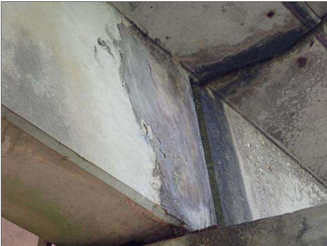
Span 5 Beam 1: WEST FACE AT BENT 4 HAS A PATCHED AREA (2 FOOT X FULL HEIGHT) THAT IS CRACKED (U TO 1/32 INCH)
