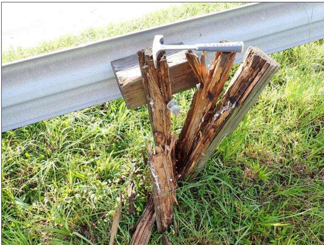
(PAR) southwest guardrail, 13th timber post from end bent 1, decay/section loss (up to full width x full height x full depth)
