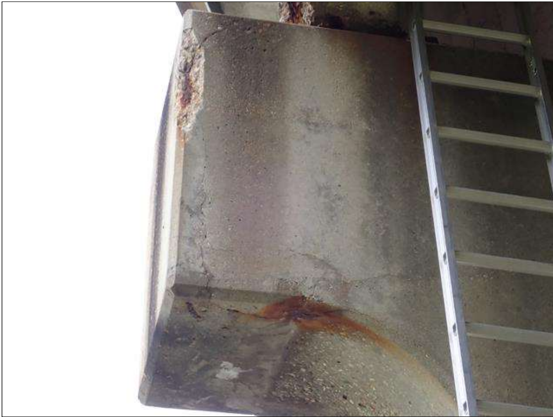
Bent 2 Cap 1: (PAR) southwest corner, spall/delamination (18 inch x 6 inch x 1 inch deep) with exposed rusted rebar and adjacent map cracks (up to 1/32 inch) with rust stains
