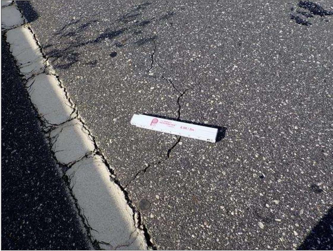
Span 5 Wearing Surface: WEARING SURFACE HAS SCATTERED TRANSVERSE AND LONGITUDINAL CRACKS UP TO 1/8 INCH
