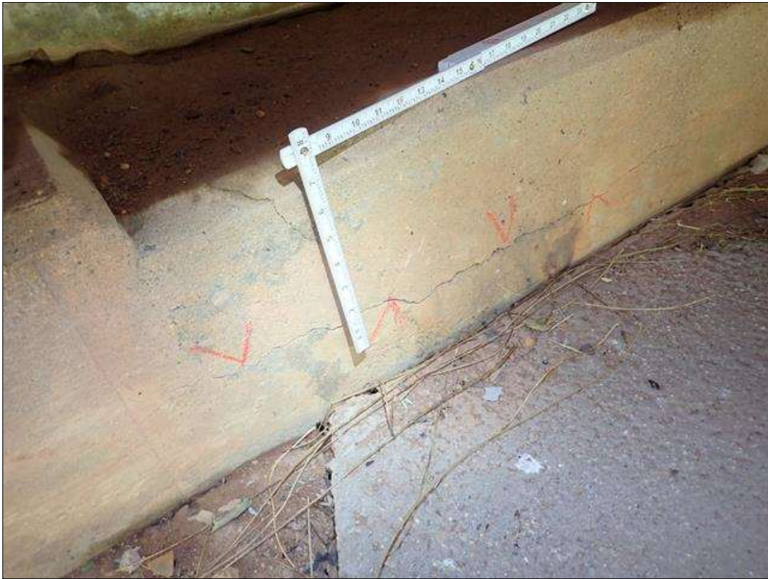
End Bent 2 Cap 1: in bay 1, horizontal crack (1/8 inch x 2.5 foot)
