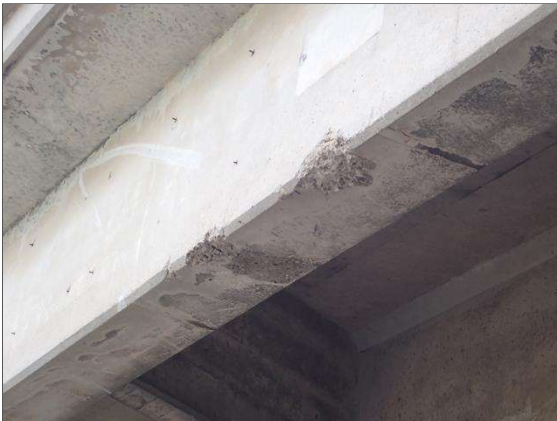
Span 4 Beam 4: EAST FACE AND BOTTOM OVER WEST BOUND RIGHT LANE. (2) 8 INCH LONG X 6 INCH X 1.5 INCH DEEP SPALLS IN MID-SPAN FROM PREVIOUS IMPACT DAMAGE.
