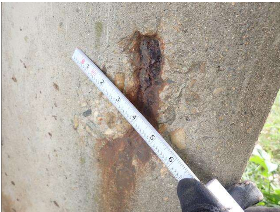
Bent 3 Pile 1: (PAR) 6 INCH DIAMETER X 1/2 INCH SPALL WITH EXPOSED REINFORCING (APPROXIMATELY 10 PERCENT LOSS) ON EAST FACE NEAR GROUNDLINE.
