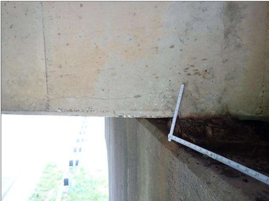
Span 4 Beam 3: near bent 3, west and east faces, longitudinal cracks (up to 1/32 inch x 2 foot)
