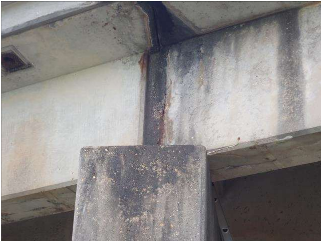
Span 4 Beam 4: (PAR) at bent 3, east face, spall/delamination (43 inch x 43 inch x 1 inch deep) with exposed rusted rebar (approximately 25 percent loss) and cracks (up to 1/32 inch)
