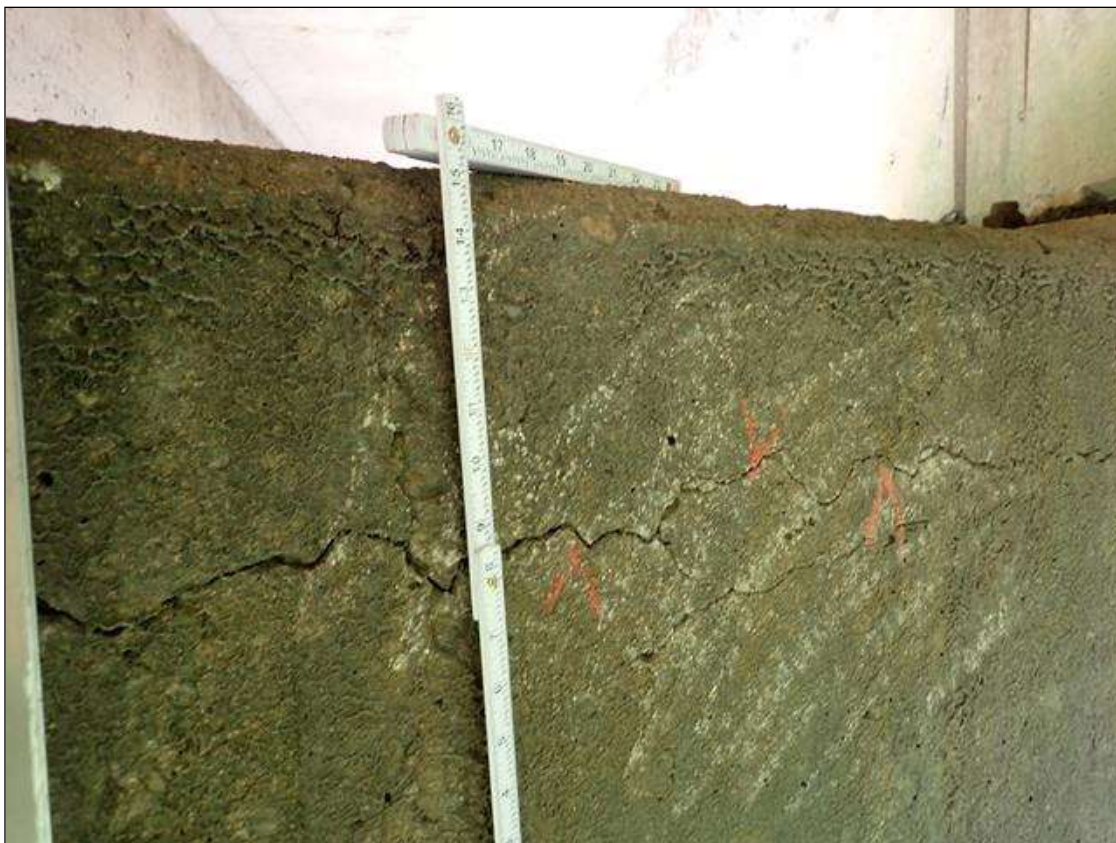
Bent 4 Cap 1: BENT 4 CAP HAS SCATTERED VERTICAL AND LONGITUDINAL CRACKS UP TO 1/16 INCH
