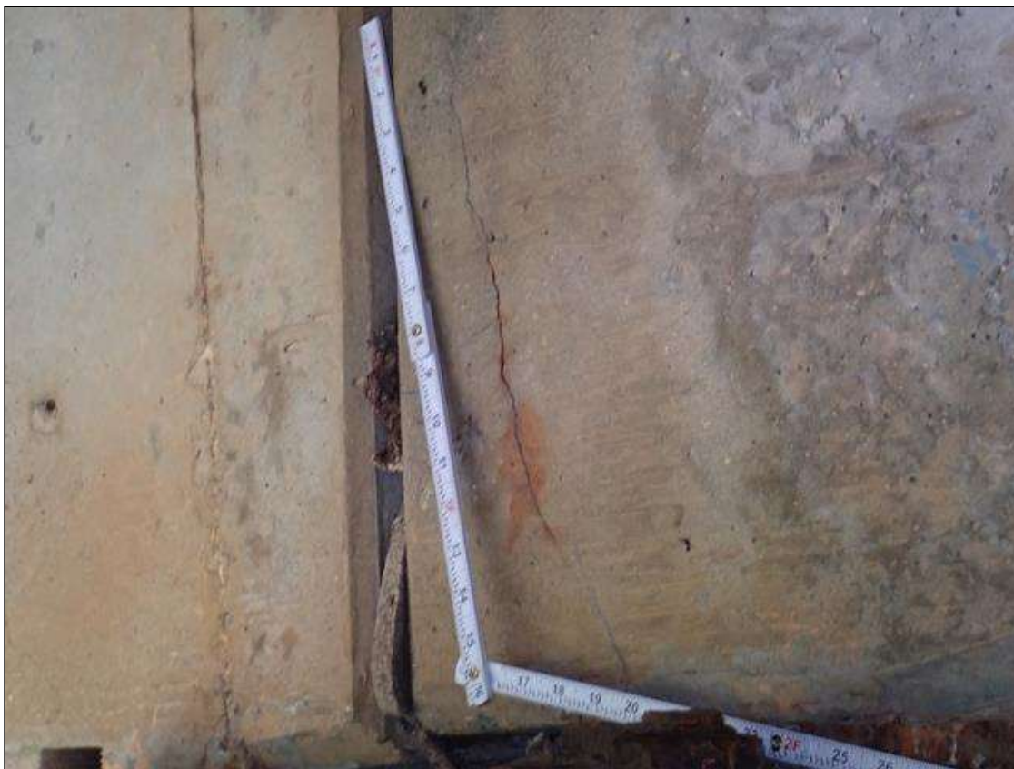
Span 1 Beam 3: (PAR) West face at far end, diagonal crack [18 inch x 1/32 inch] with rust stain
