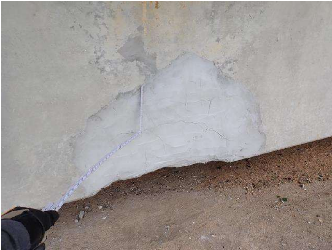
Span 5 Beam 4: 2023 previously repaired with patch (3.5 foot x 2.5 foot) with map cracks (up to 1/32 inch), previously noted as: lower East face at 12 foot from end bent 2, spall [40 inch long x 26 inch high x up 5 inch deep] with exposed primary rebar and stirrups, section loss on rebar [up to 1/16 inch]
