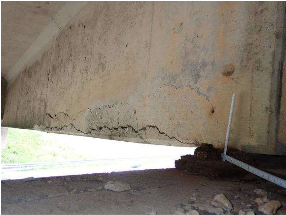
Span 3 Beam 4: (PAR) West face at near end, delamination [11 foot long x up to 9 inch high] with associated 1/2 inch crack, delamination extends to right Eastbound lane of I-40 below
