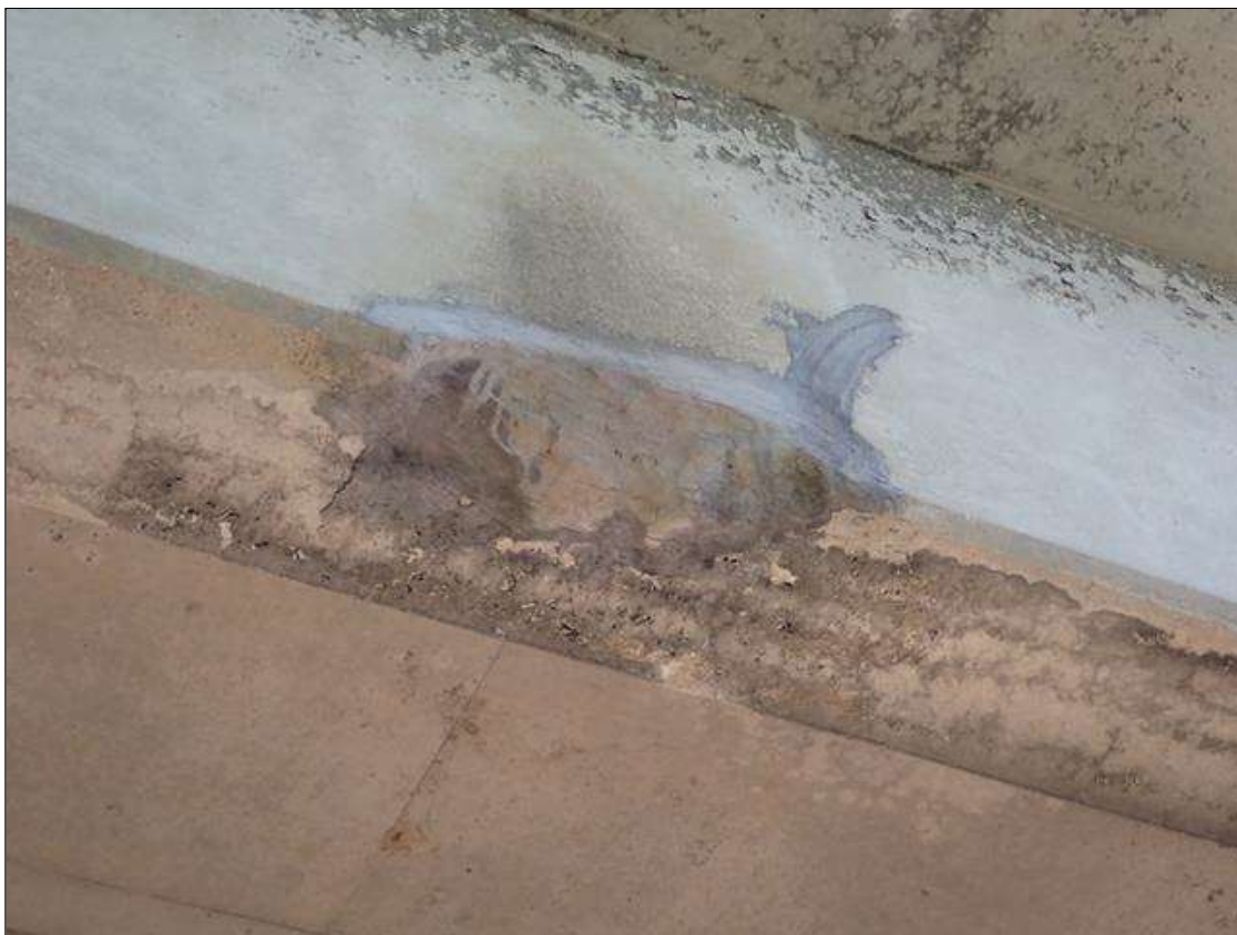
Span 4 Beam 1: WEST FACE AND BOTTOM HAS A PATCHED AREA (2.5 FOOT X 1.5 FOOT) WITH HAIRLINE MAP CRACKING.
