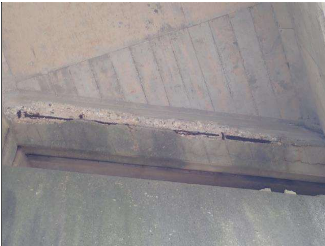
Span 3 Beam 1: (PAR) at bents 2 and 3, bay 1 end diaphragms, spalls/delaminations (up to full length x full height x up to 1.5 inch deep) with exposed rusted rebar (approximately 25 percent loss) and cracks (up to 1/8 inch)
