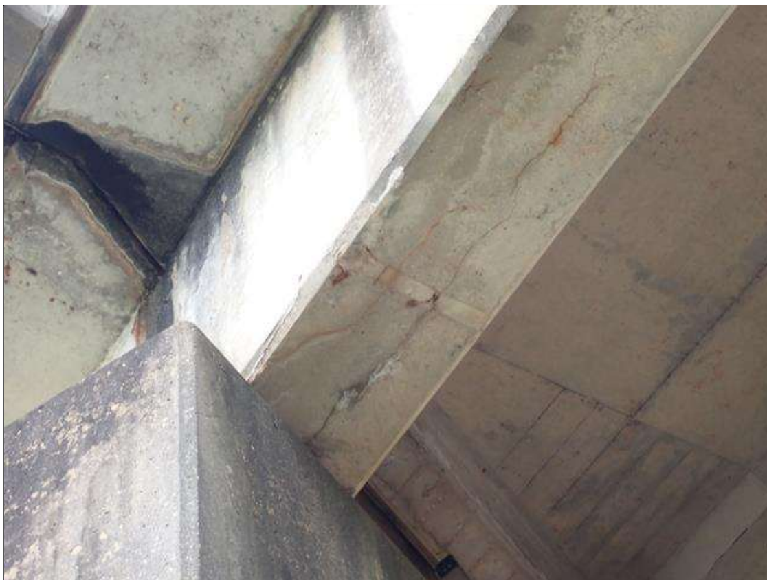
Span 4 Beam 4: (PAR) AT BENT 3, (2) UP TO 7 FOOT X 1/32 INCH LONGITUDINAL CRACKS, ON BOTTOM AND WEST FACES WITH EFFLORESCENCE AND RUST STAIN
