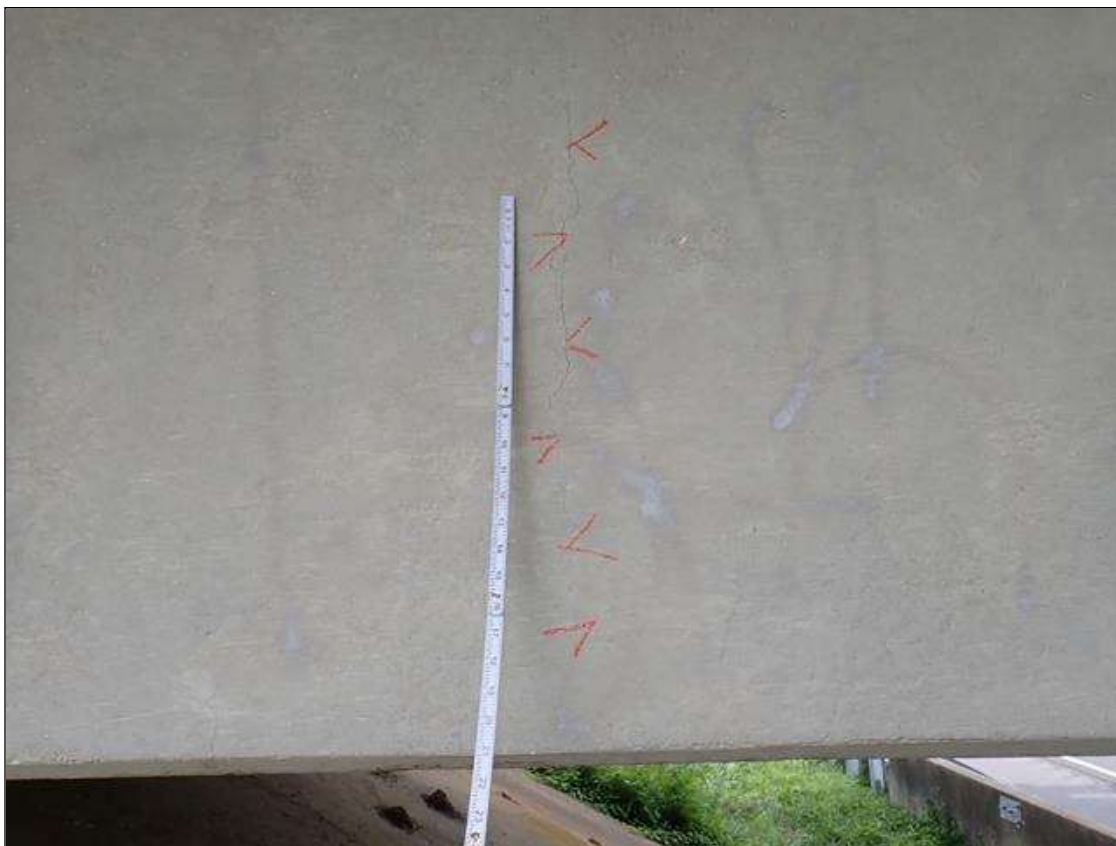
Span 5 Beam 1: TRANSVERSE AND WRAPAROUND CRACKS UP TO 1/64 INCH, AT RANDOM THROUGHOUT.
