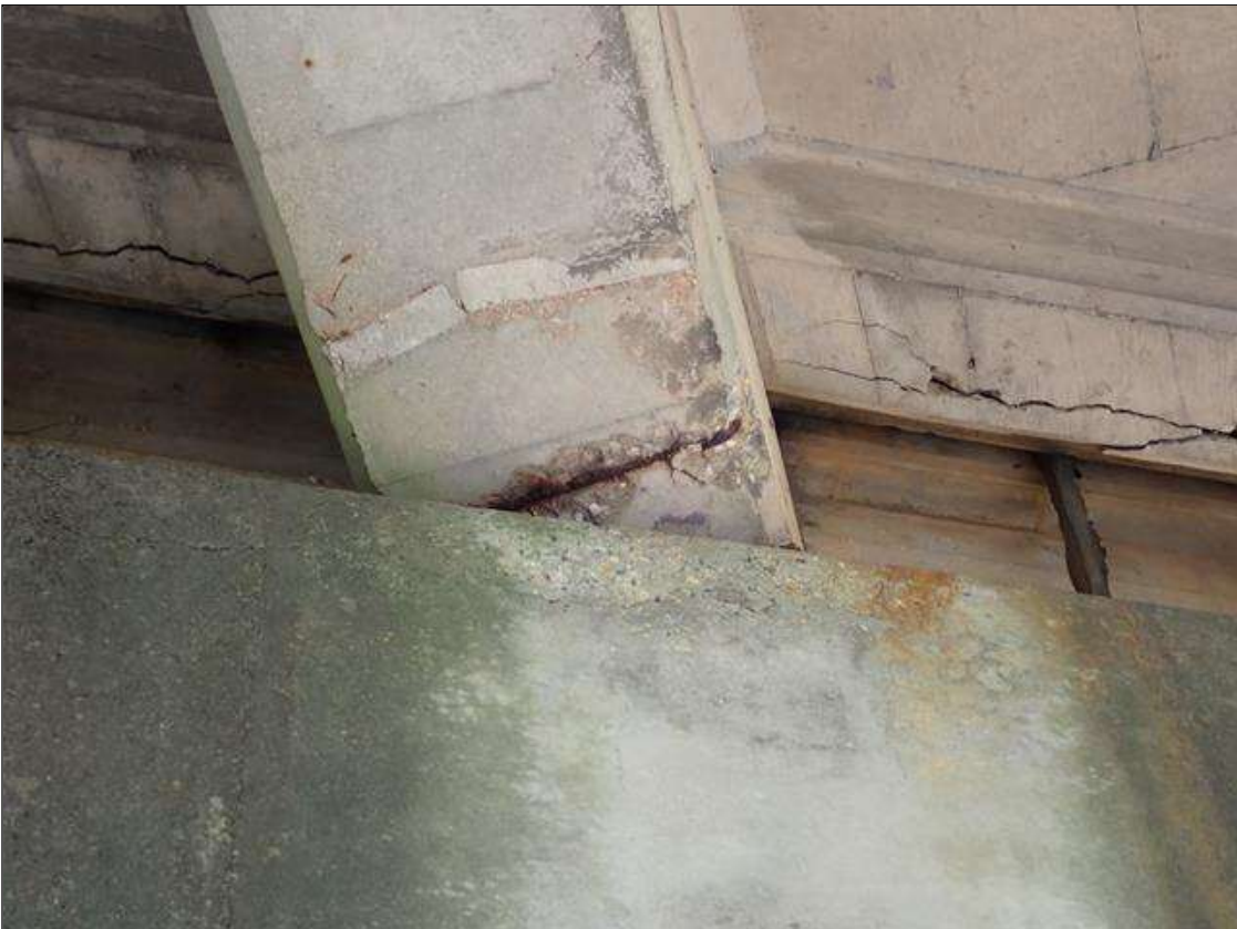
Span 4 Beam 2: BOTTOM OF BEAM 2 OVER BENT 4. HAS A CRACK/SPALL AND DELAMINATED AREA WITH REBAR EXPOSED. AREA IS: 8 INCH X FULL WIDTH X 1/2 INCH DEEP [NO LOSS NOTED]
