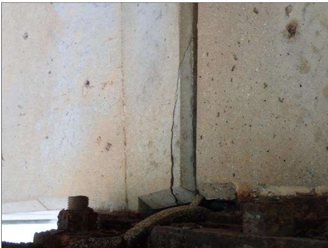
Span 3 Beam 3: at bent 2, west face, delamination (2 inch x 1 foot) with cracks (up to 1/8 inch)
