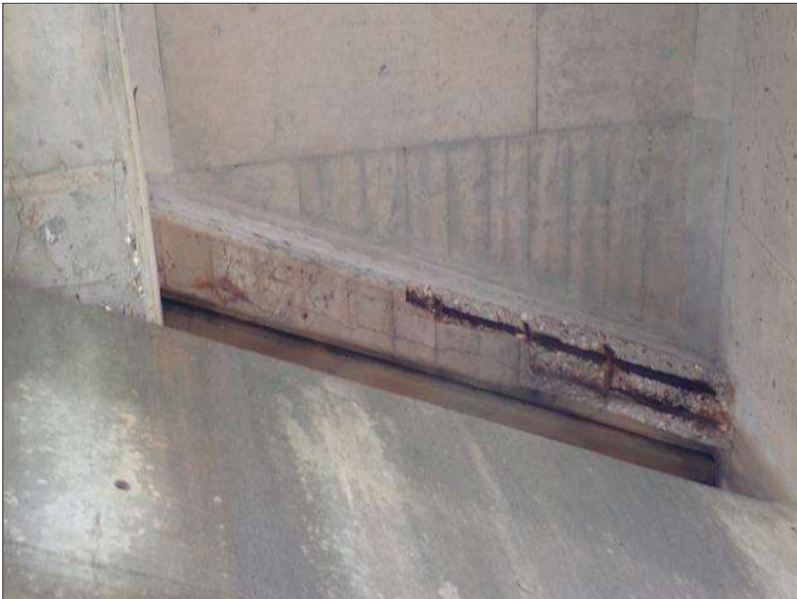
Span 4 Beam 2: (PAR) at bents 3 and 4, bay 2 end diaphragms, spalls/delaminations (up to full length x full height x up to 1.5 inch deep) with exposed rusted rebar (approximately 25 percent loss) and cracks (up to 1/8 inch) with rust stains
