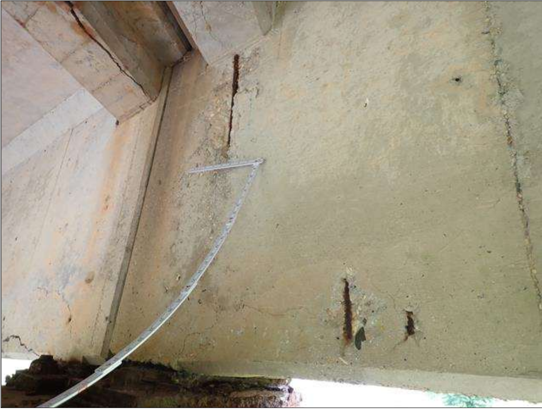
Span 2 Beam 4: (PAR) at bent 2, west and east faces and underside, multiple spalls/delaminations (up to 18 inch x 8 inch x 1 inch deep) with exposed rusted rebar (approximately 25 percent loss)
