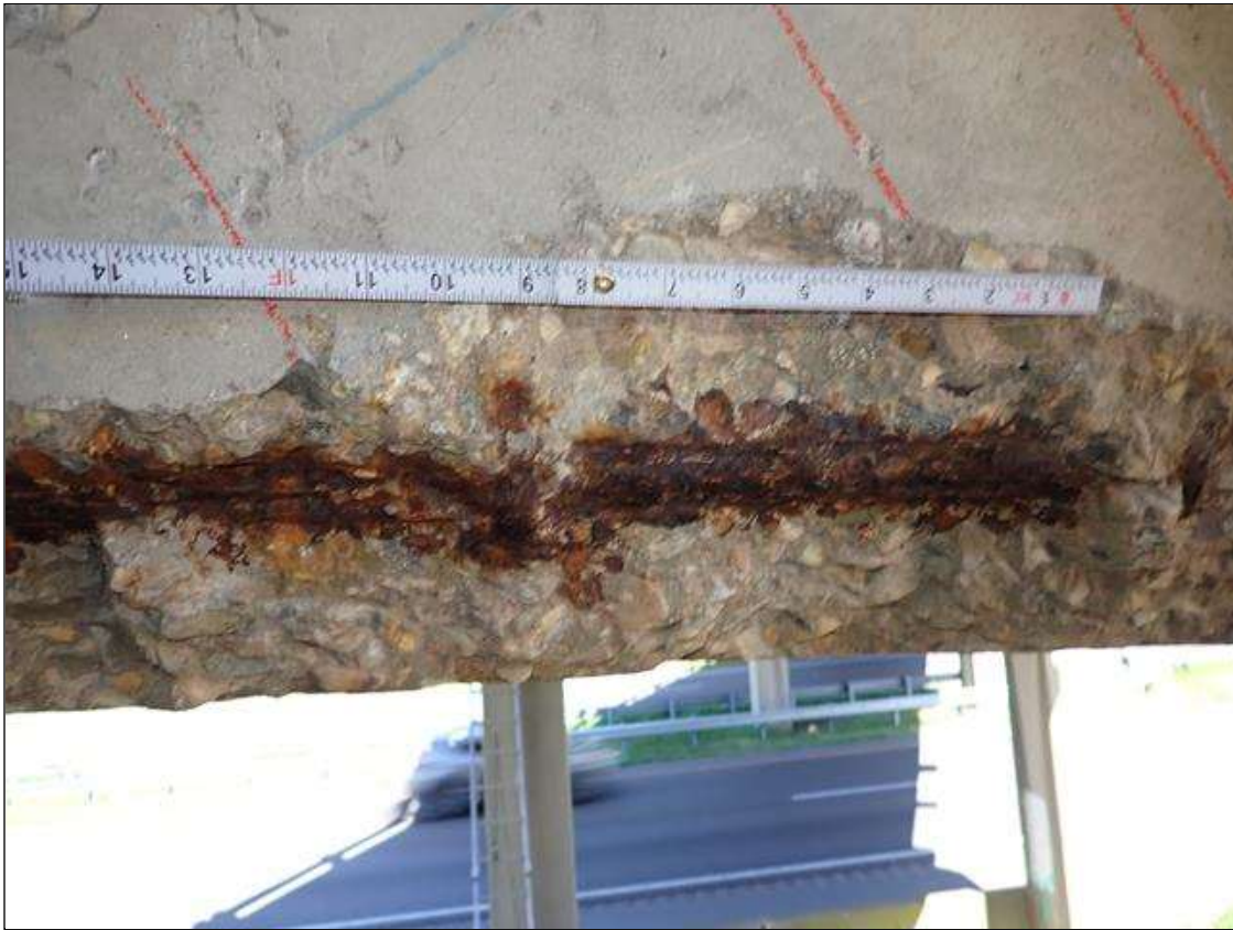
Bent 1 Cap 1: (PAR) along north and south faces, multiple spalls/delaminations (up to 16 foot x full height x 2.5 inch deep) with exposed rusted rebar (approximately 25 percent loss) and cracks (1/8 inch) at random
