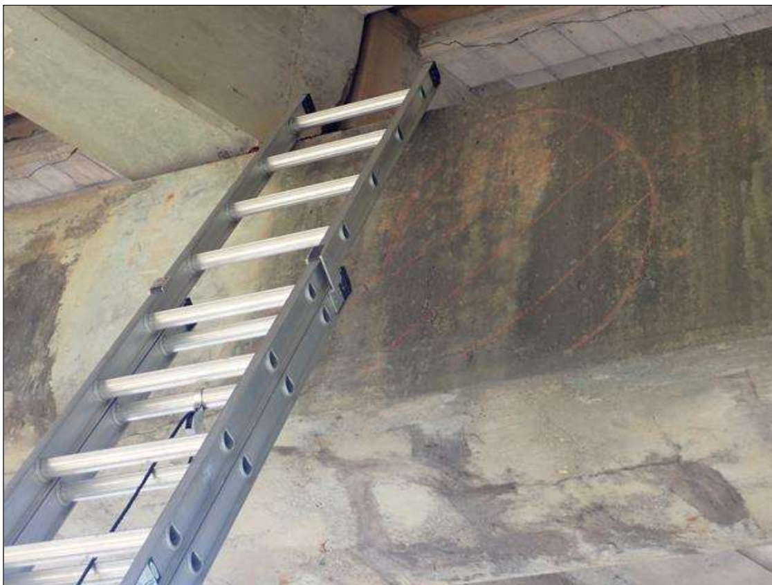
Bent 4 Cap 1: NORTH FACE BAY 2. HAS A CRACKED AND DELAMINATED AREA [UP TO FULL HEIGHT X 5.5 FOOT]
