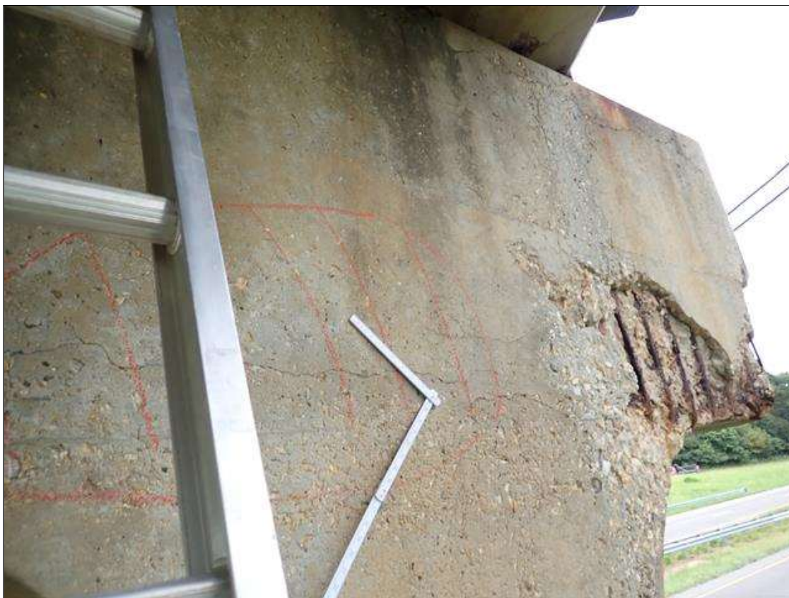
Bent 2 Cap 1: (PAR) South face at East end, spall/delamination [84 inch long x up to full height x up to 3 inch deep] with exposed rusted rebar and stirrups [rebar and stirrups with approximately 25 percent loss] and cracks [up to 1/8 inch]
