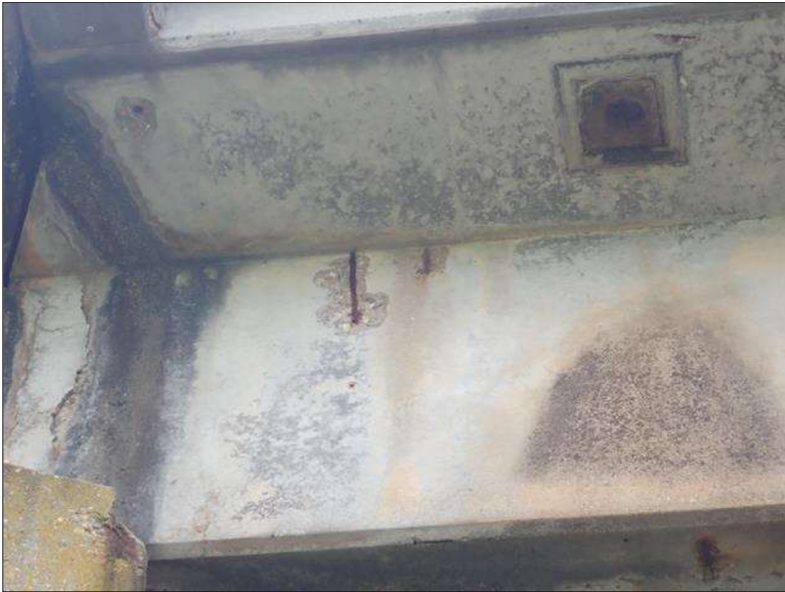
Span 3 Beam 4: EAST FACE. HAS (2) AREAS THAT ARE SPALLED WITH REBAR EXPOSED. LOCATED 38 INCH FROM END OF BEAM OVER BENT 2. AREAS ARE: UP TO 8 INCH X 14 INCH X 3/4 INCH DEEP.
