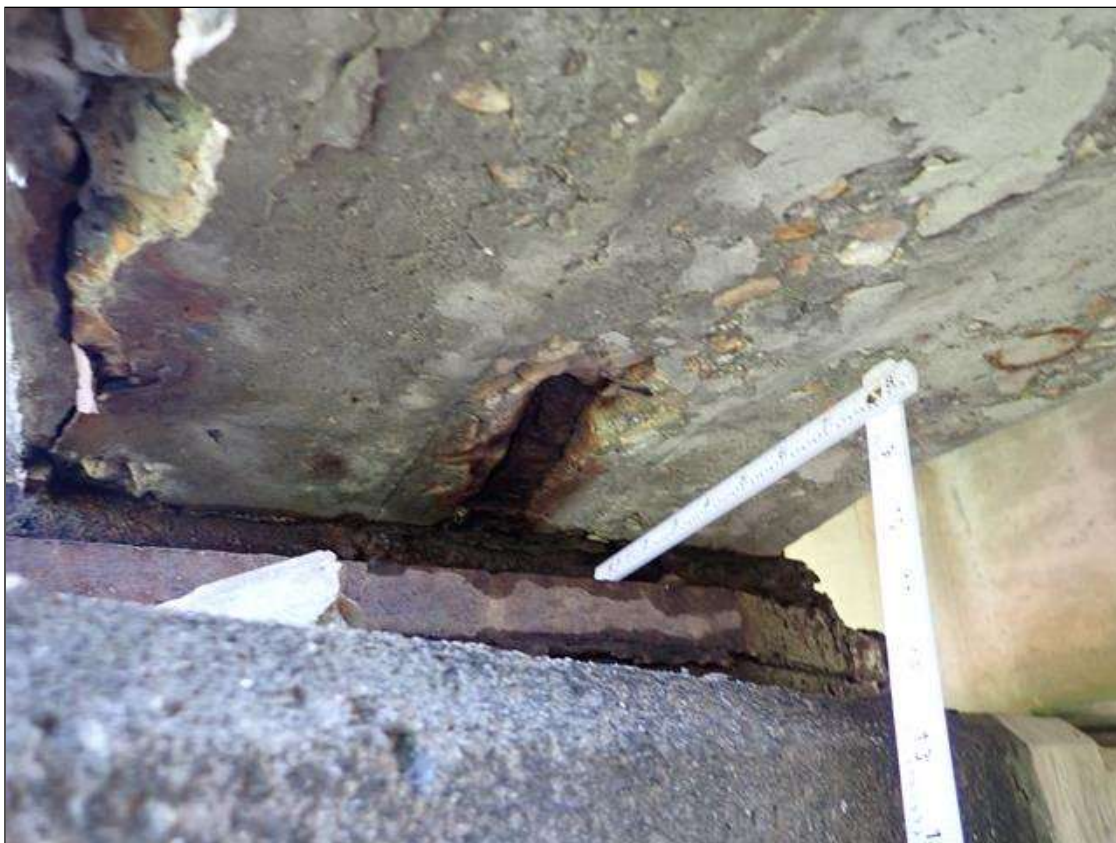
Span 1 Beam 1: (PAR) at bent 1, west face and underside, (2) spalls/delamination (up to 2.5 foot x 2 foot x 2 inch deep) with exposed rusted rebar (approximately 25 percent loss)
