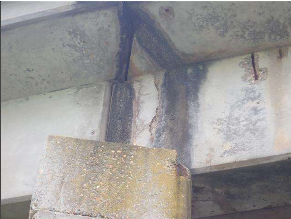
Span 3 Beam 4: EAST FACE OVER BENT 2. HAS A SPALL WITH ADJACENT DELAMINATED AREA 7 INCH FROM END OF BEAM. AREA IS: 10 INCH X 30 INCH X 1/2 INCH DEEP.
