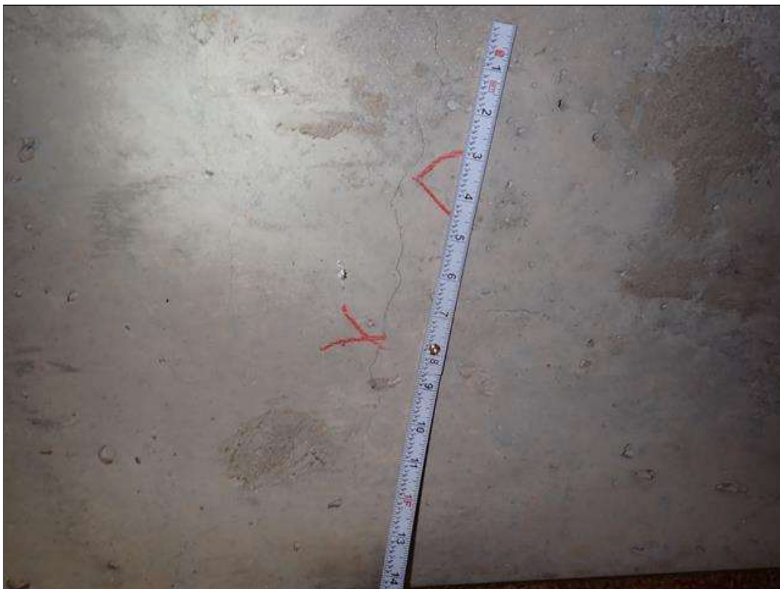
Span 1 Beam 3: along far half of beam, vertical/diagonal cracks (up to 1/64 inch x full height)
