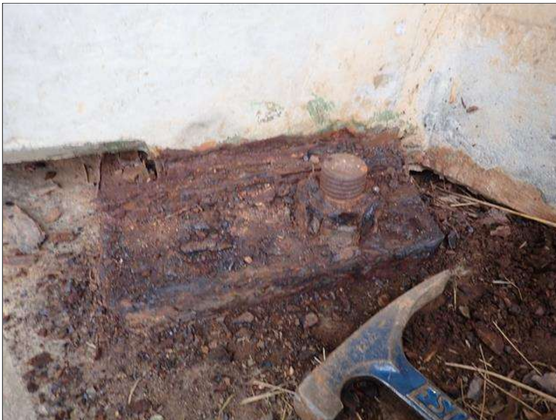
Span 5 Far Bearing 4: corrosion with section loss [up to 3/16 inch loss]
