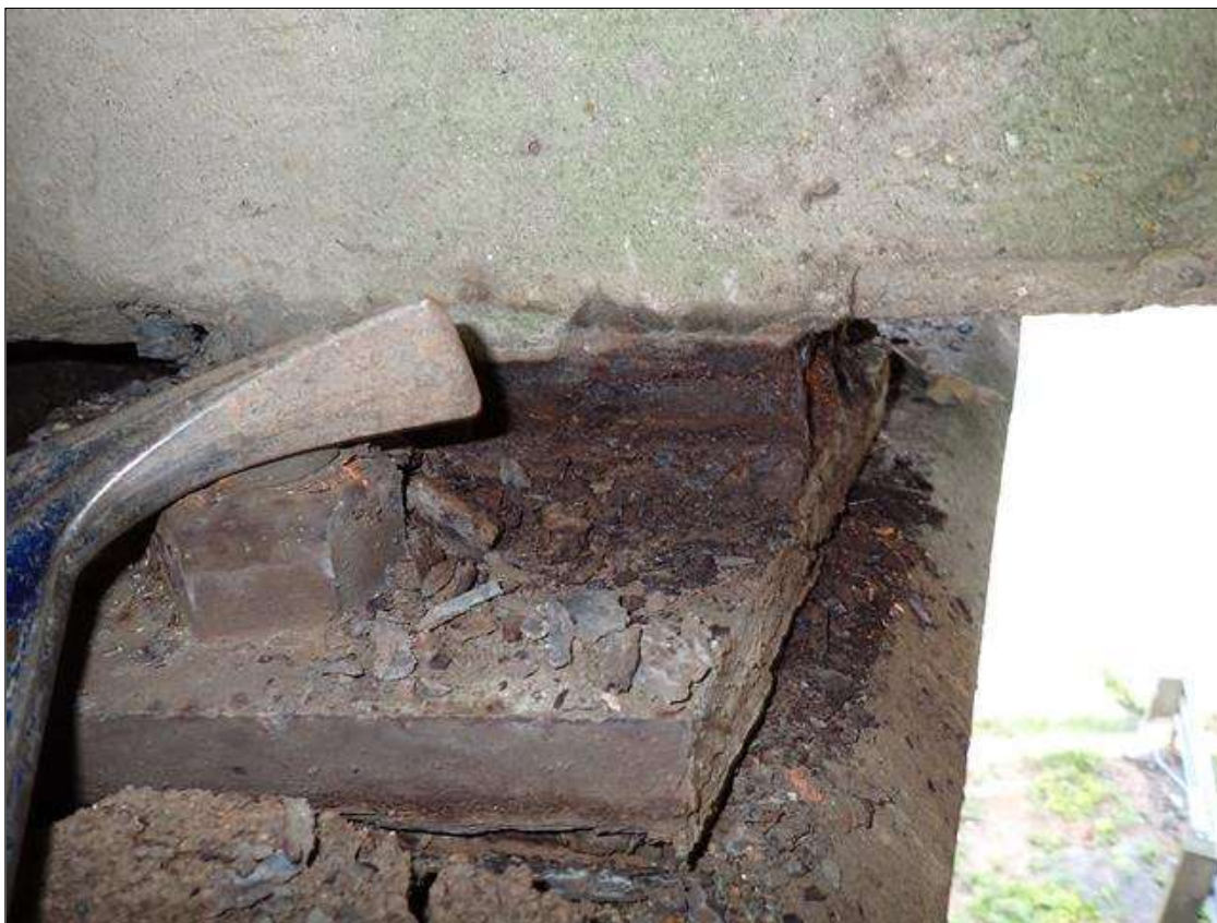
Span 3 Beam 4 - Far Bearing 4: corrosion with section loss (up to 1/8 inch)
