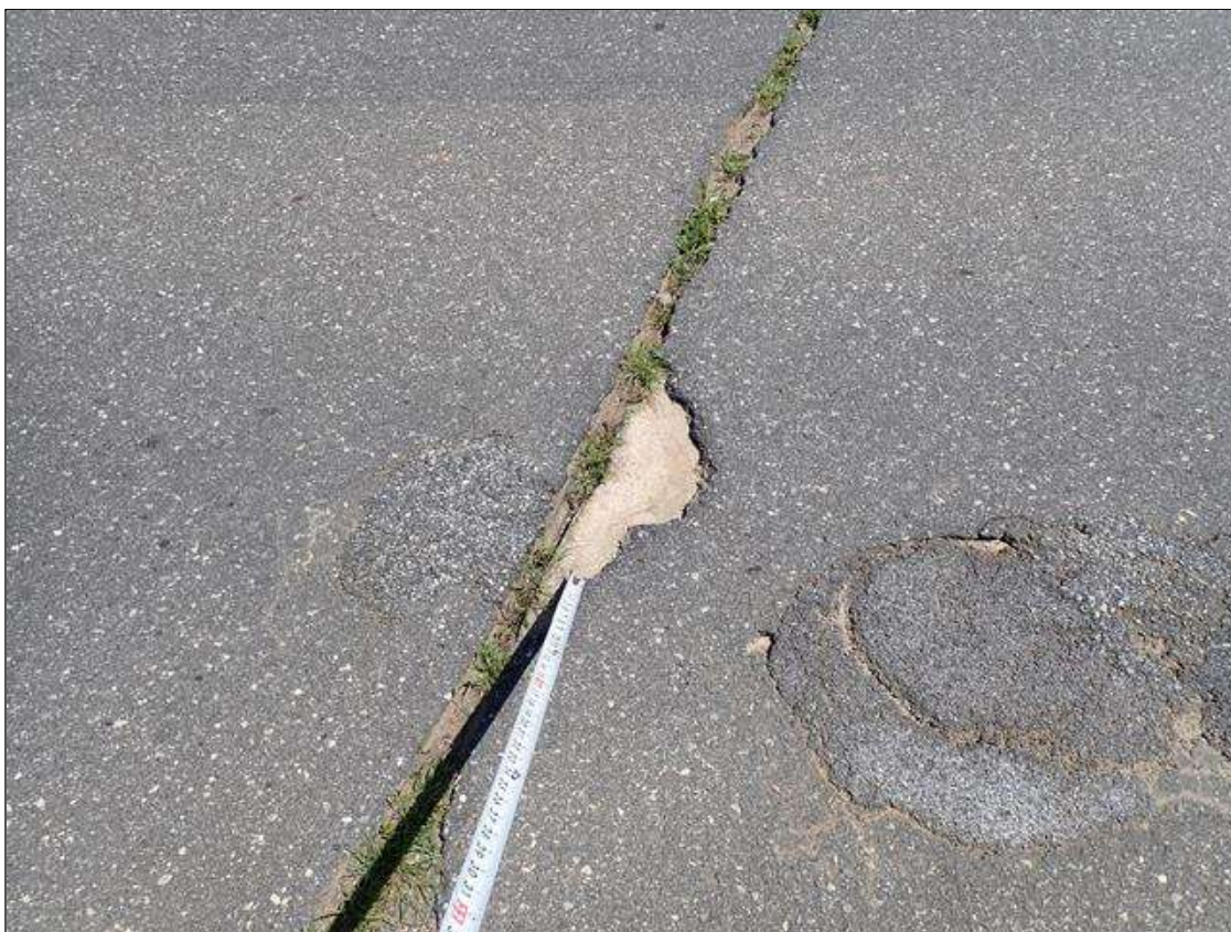
Span 3 Wearing Surface: (PAR) at bent 3, southbound lane, pothole (2 foot x 9 inch x full depth)
