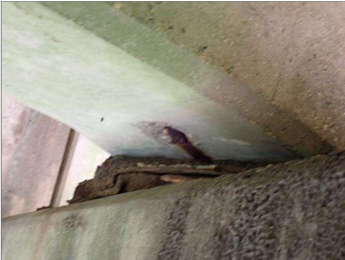
Span 2 Beam 2: at bent 2, underside, spall (6 inch x 3 inch x 1/2 inch deep) with exposed rusted rebar
