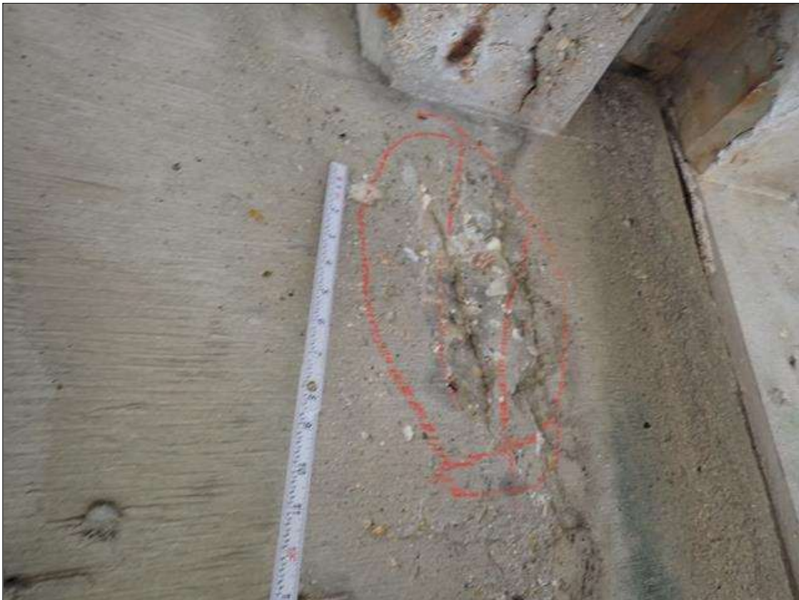
Span 3 Beam 1: at bent 3, east face, spall/delamination (8 inch x 12 inch x 1/2 inch deep); underside, spall (4 inch x 3 inch x 1/2 inch deep) with exposed rusted rebar
