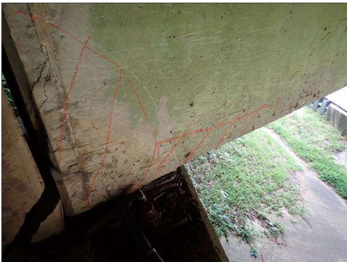
Span 2 Beam 1: east face at bent 1, delamination (32 inch x 18 inch) with cracks (up to 1/32 inch)
