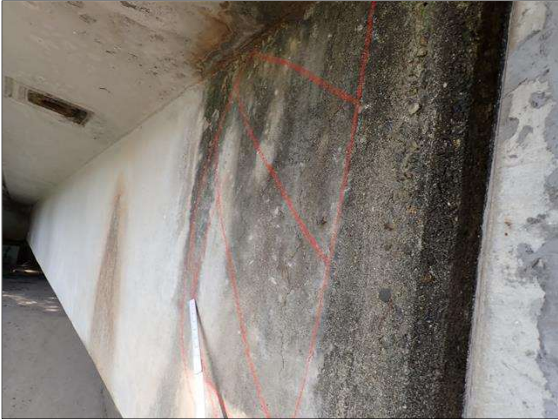
Span 5 Beam 1: SPAN 5 BEAM 1 WEST FACE WEB OVER BENT 4. HAS A CRACKED AND DELAMINATED AREA. AREA IS: 24 INCH X 32 INCH
