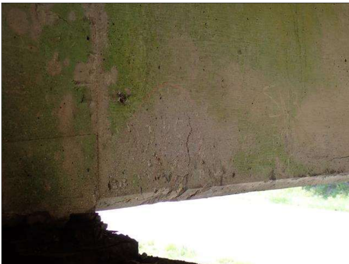
Span 3 Beam 1: east face web at bent 2, delamination [12 inch x 10 inch]
