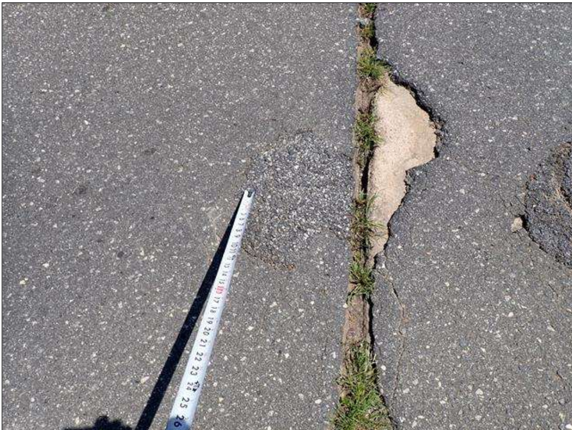
Span 4 Wearing Surface: 1 FOOT DIAMETER PATCH SOUTHBOUND LANE BENT 3.
