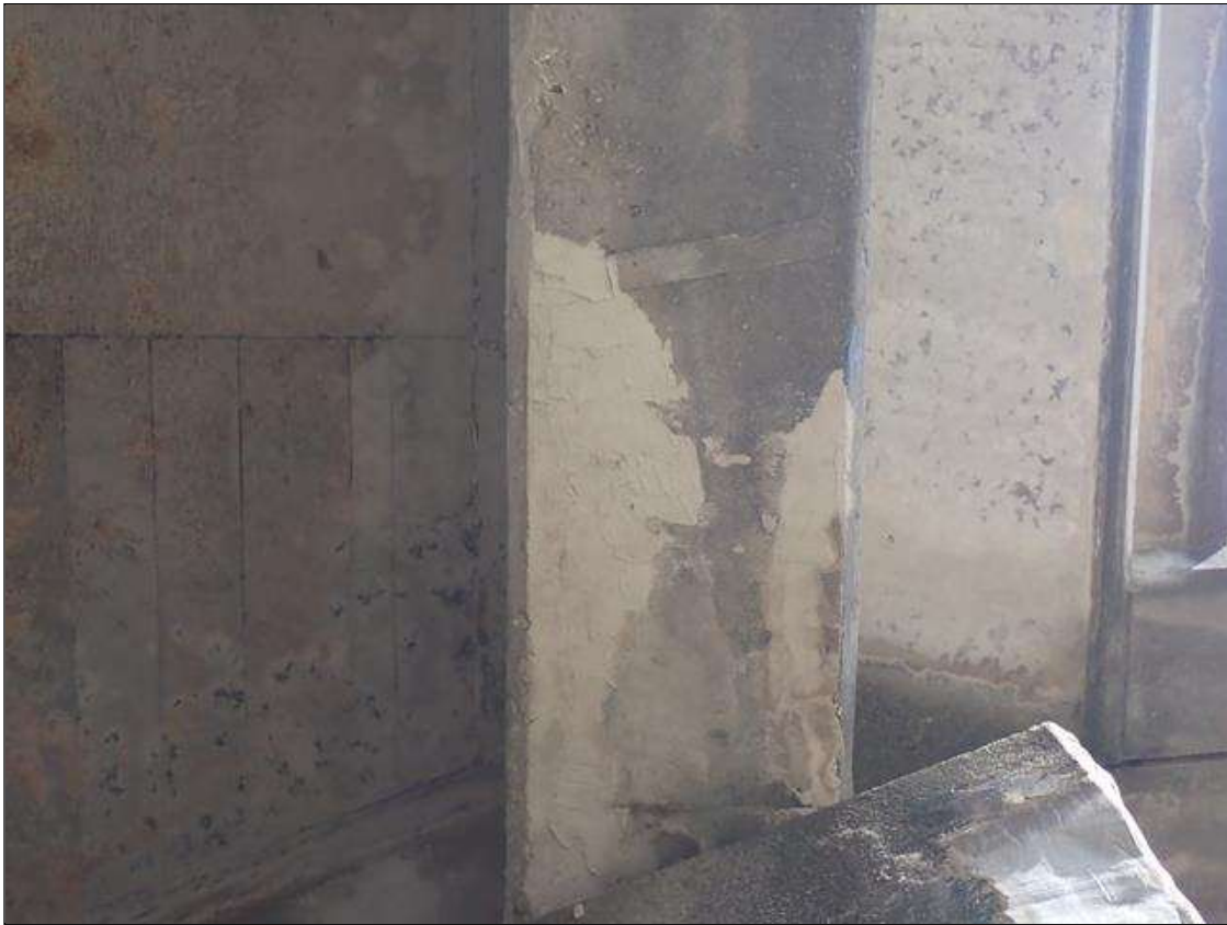
Span 4 Beam 1: 2023 NEW REPAIR, PATCHED AREAS (UP TO 2.5 FOOT X FULL WIDTH), PREVIOUSLY NOTED AS: LONGITUDINAL CRACKS [UP TO 3 FOOT X UP TO 1/8 INCH] ON BOTTOM FACE AT BENT 3 WITH ASSOCIATED DELAMINATION THAT WRAPS AROUND TO EAST FACE [3 FOOT X 5 FOOT]
