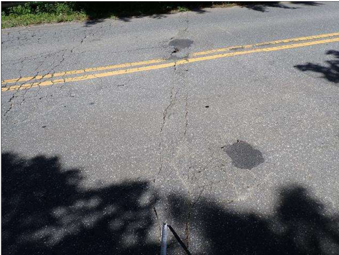
Span 1 Wearing Surface: along length of asphalt over end bent 1, transverse cracks [up to 1/4 inch x full roadway width] with edge spalling up to (1/2 inch deep) and associated sound patch [4 foot x 8 inch]
