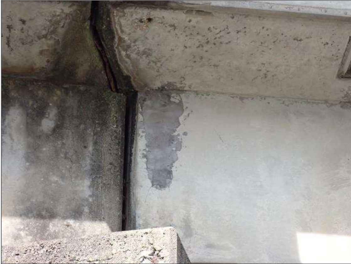
Span 4 Beam 1: 2023 PREVIOUSLY REPAIRED, PATCHED AREA, PREVIOUSLY NOTED AS: SUPPLEMENTAL INSPECTION IMPACT DAMAGE 2021 : 9 INCH X 14 INCH X 3/4 INCH SPALL WITH EXPOSED RUSTED REINFORCING NO SECTION LOSS WEST FACE AT BENT 4
