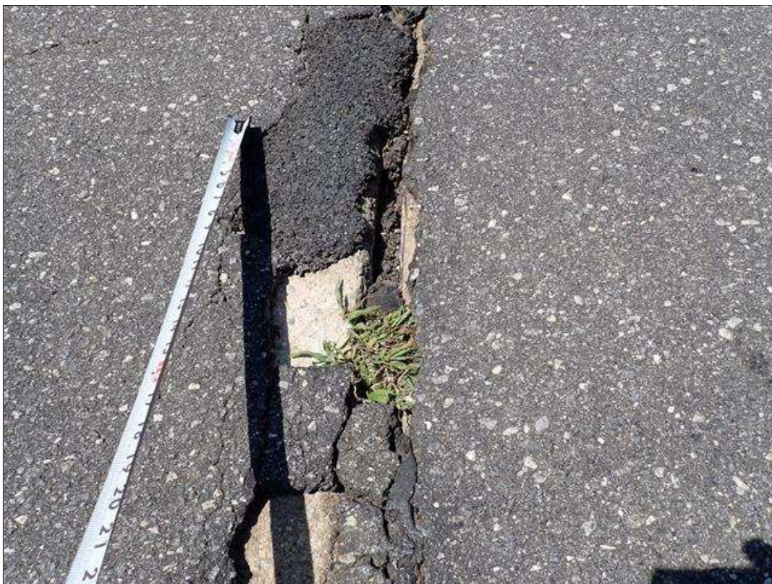
Span 3 Expansion Joint 2: along the length of the joint, joint material deteriorated/torn/missing at random
