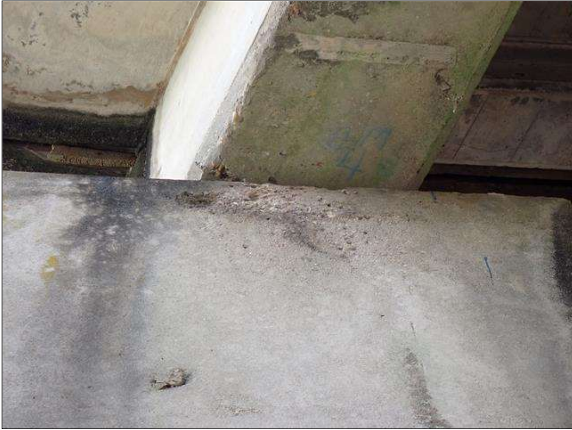
Bent 3 Cap 1: north face under beam 4 delamination [2.5 foot x 1.5 foot] with associated map cracking [up to 1/64 inch] and honeycombing
