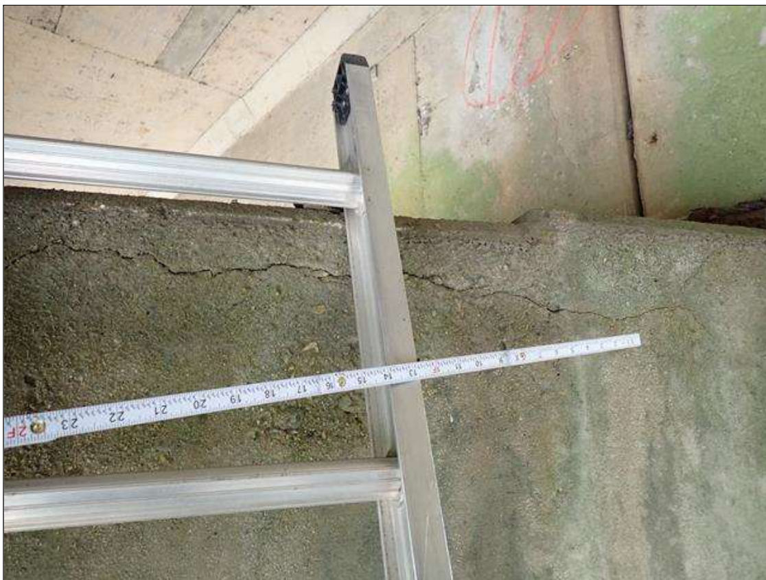
Bent 3 Cap 1: along the length of the cap, vertical cracks (up to 1/64 inch x full height) and longitudinal cracks (up to 1/32 inch x 6 foot) at random
