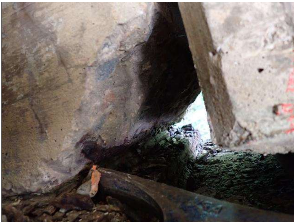
Span 1 Beam 1: (PAR) at bent 1, east face, bottom of beam, spall (full width x 5 inch x 2 inch deep) with exposed rusted rebar (approximately 25 percent loss)
