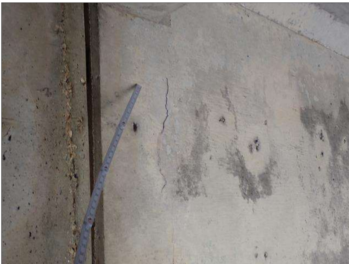
Span 4 Beam 4: at bent 4, west face, delamination (3 inch x 16 inch)
