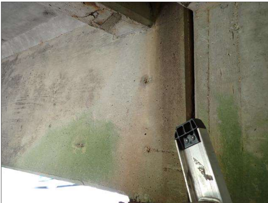
Span 4 Beam 3: (not found 2023) SUPPLEMENTAL INSPECTION IMPACT DAMAGE 2021 : SPALL AT FAR END ABOVE interior. BENT 4 , 4 INCH LONG X 4 INCH WIDE X 1 INCH DEEP.
