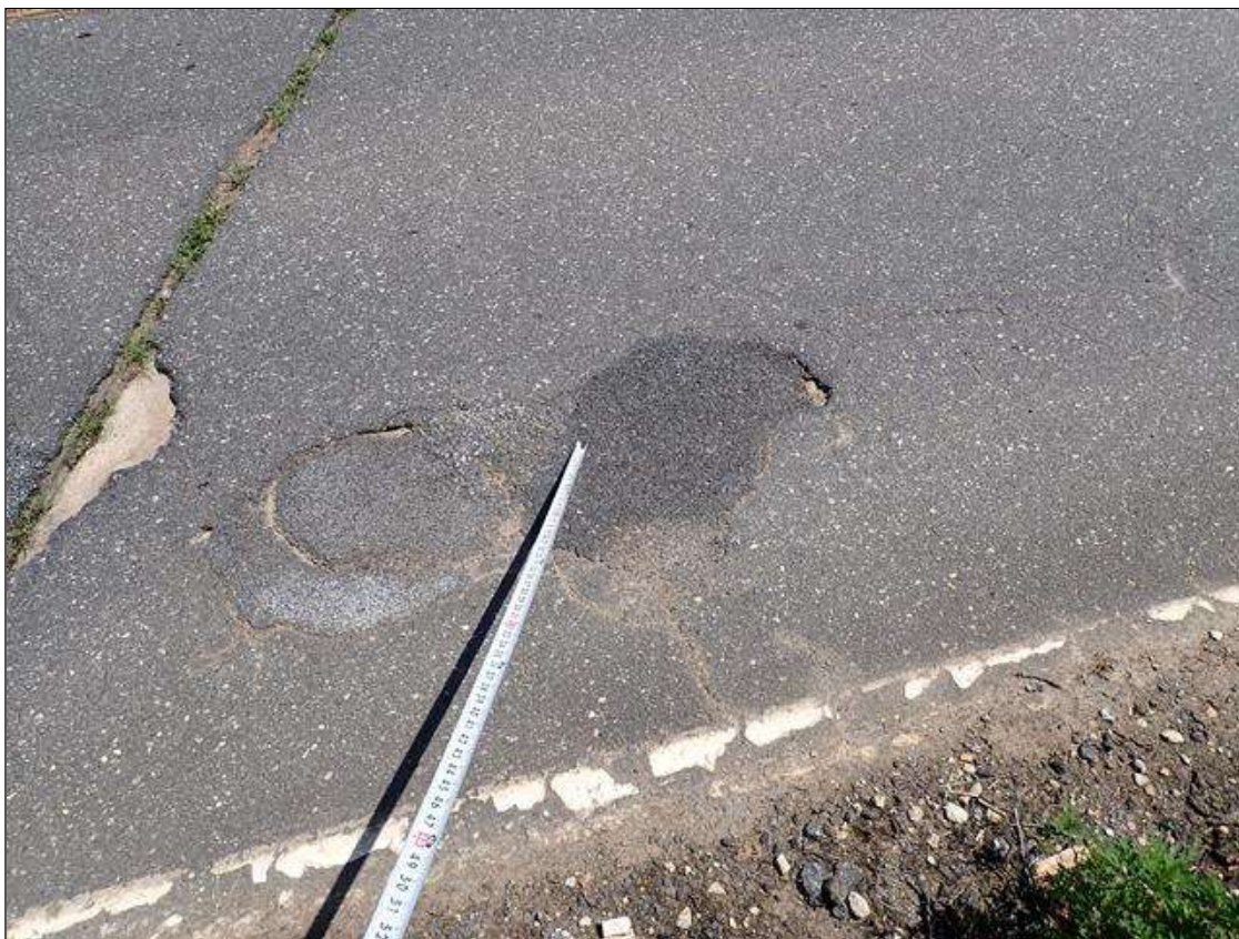
Span 3 Wearing Surface: SOUTHBOUND LANE NEAR BENT 3 UNSOUND PATCHED AREA (4 FOOT X 2 FOOT) WITH CRACKING AND EDGE SPALLING (UP TO FULL DEPTH)
