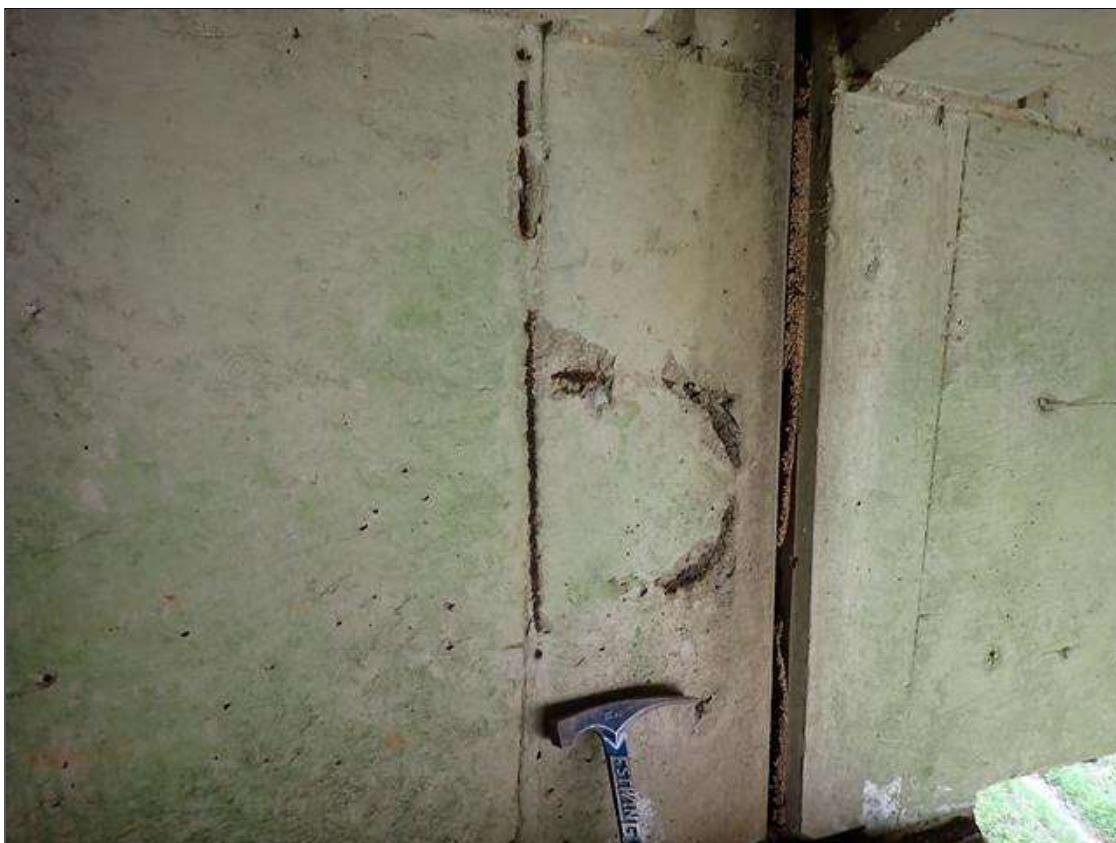
Span 1 Beam 2: east face at bent 1, multiple spalls/delaminations (up to 10 inch x 11 inch x 1/2 inch deep) with exposed rusted rebar
