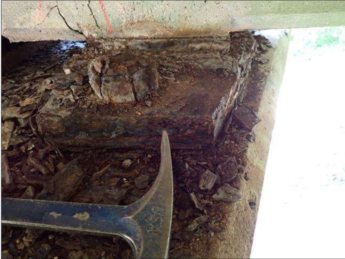
Span 1 Beam 4 - Near Bearing 4: corrosion with section loss (up to 1/8 inch deep)
