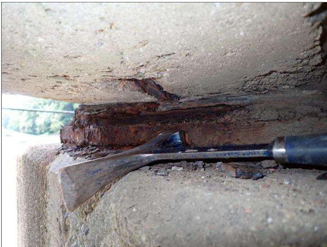
Span 3 Beam 1 - Far Bearing 1: corrosion with section loss (up to 1/16 inch)
