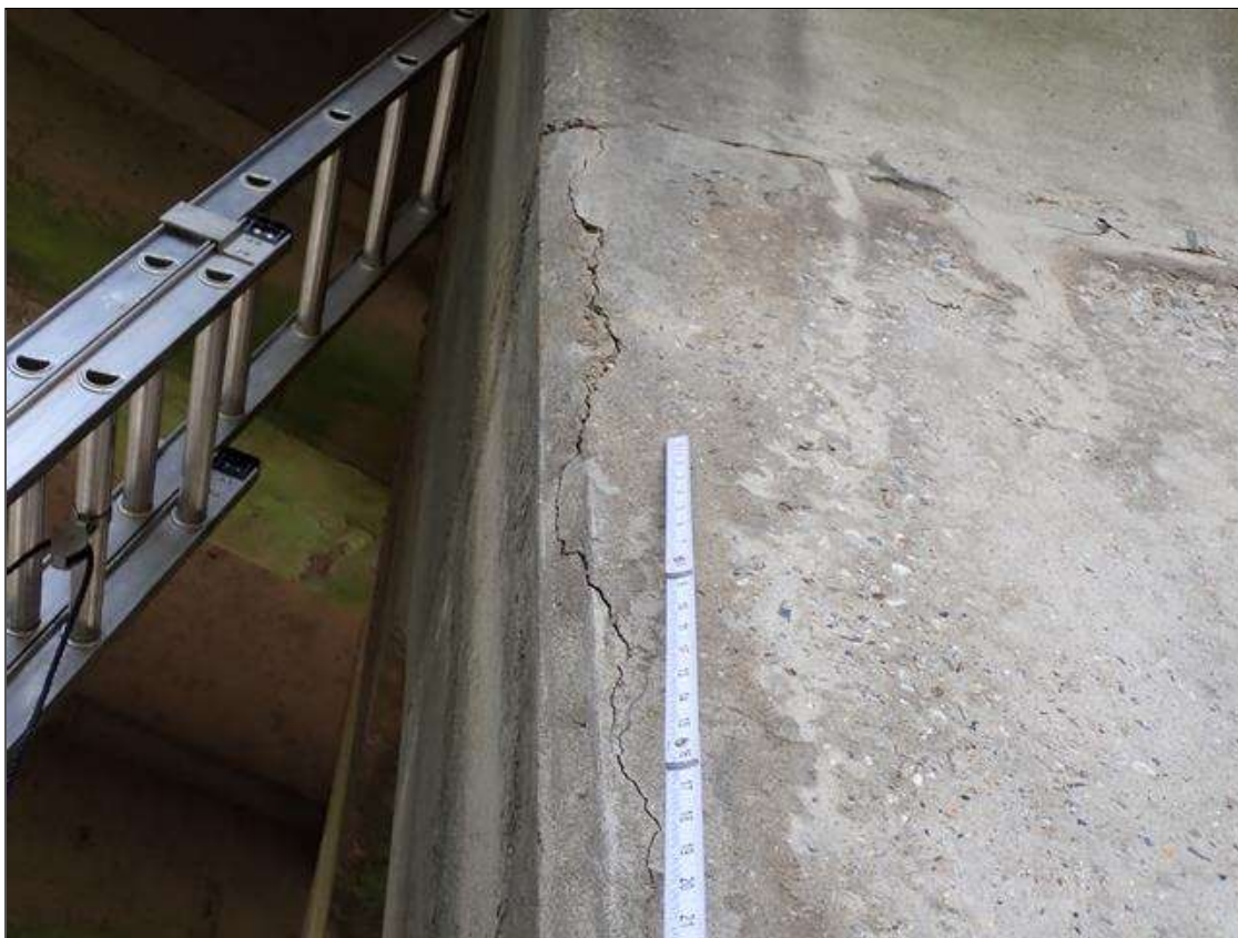
Bent 3 Pile 2: 4 FOOT X UP TO 1/16 INCH VERTICAL CRACK EAST FACE NEAR BOTTOM OF CAP
