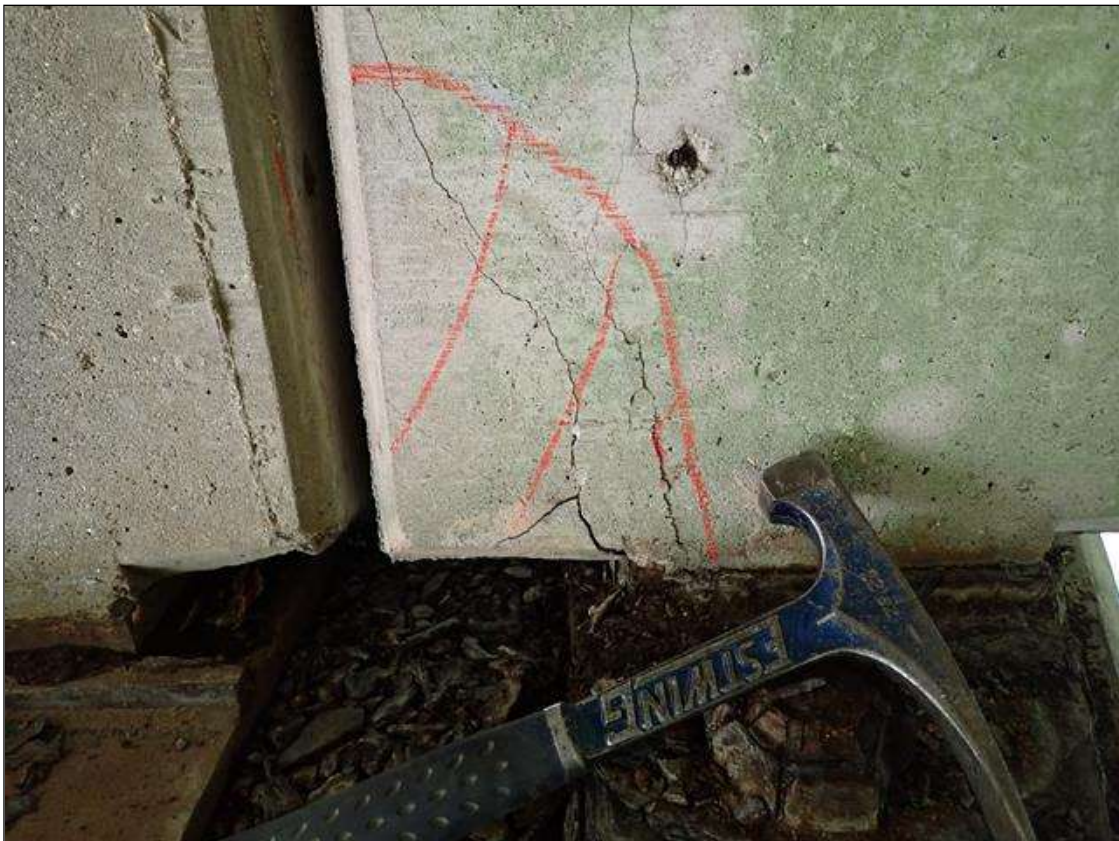
Span 1 Beam 4: at bent 1, west face, delamination (8 inch x 6 inch) with cracks (up to 1/16 inch)
