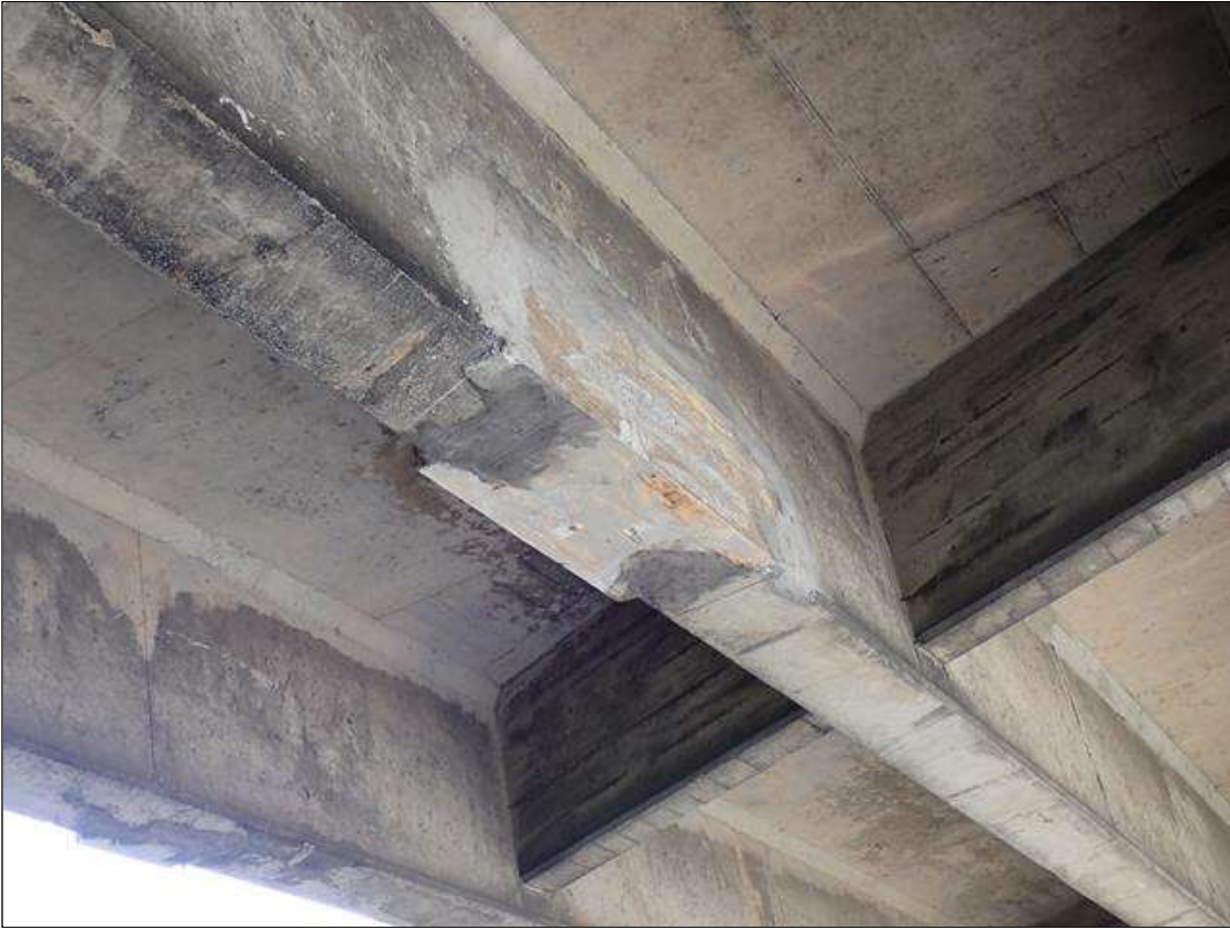
Span 4 Beam 3: 2023 NEW REPAIR, PATCHED AREA, PREVIOUSLY NOTED AS: SUPPLEMENTAL INSPECTION IMPACT DAMAGE 2021 : 4 FOOT X UP TO 10 INCH X 4 INCH SPALL WITH EXPOSED REINFORCING EAST AND BOTTOM FACE OVER WESTBOUND LANE
