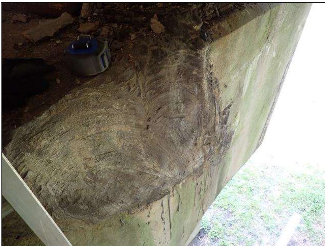
Bent 2 Cap 1: 3 FOOT X UP TO 3 FOOT PATCHED AREA SOUTH FACE UNDER BAY 3 NEAR BEAM 4
