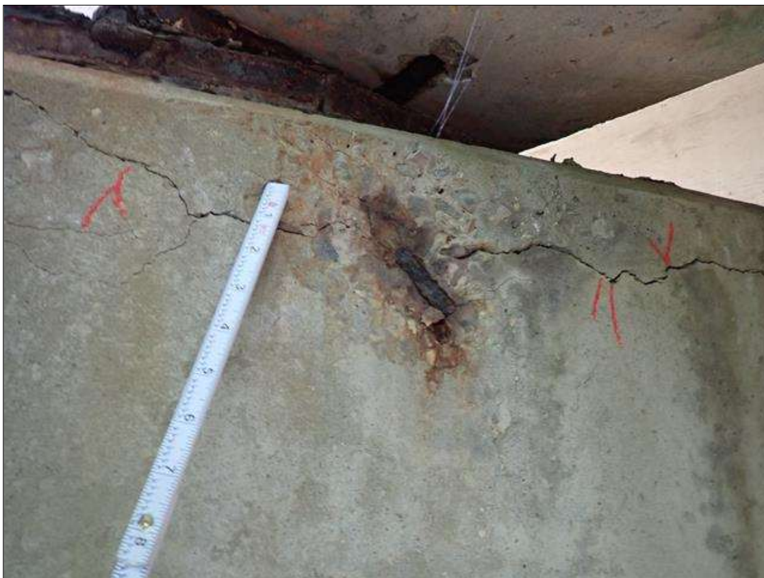
Bent 1 Cap 1: (PAR) 6 INCH DIAMETER X 1 INCH SPALL WITH EXPOSED REINFORCING APPROXIMATELY 25 PERCENT SECTION LOSS SOUTH FACE UNDER BEAM 1
