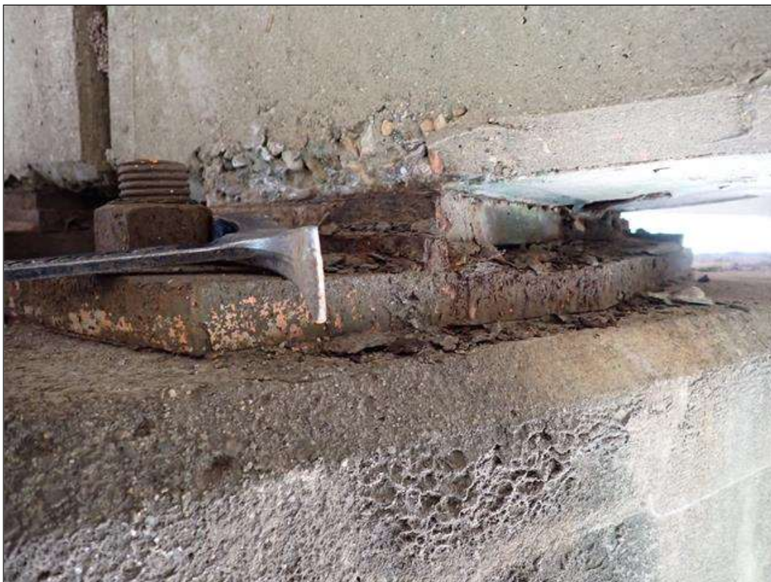
Span 5 Beam 2 - Near Bearing 2: surface rust/rust scale
