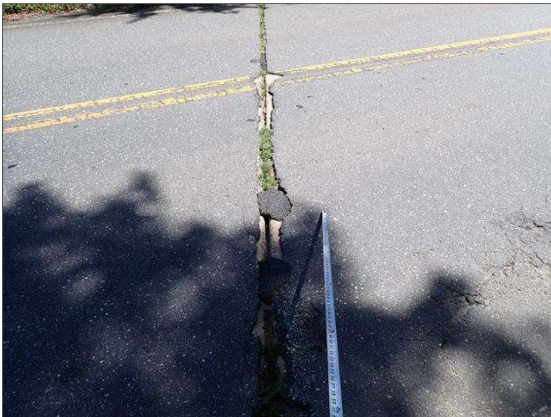
Span 1 Wearing Surface: (PAR) at bent 1, southbound lane, partially patched pothole (13 foot x 6 inch x full depth)
