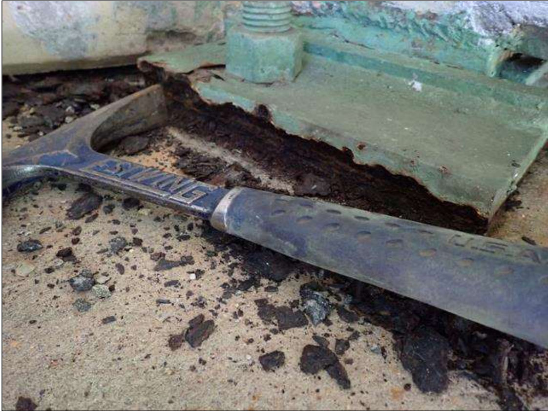
Span 1 Beam 4 - Near Bearing 4: corrosion with section loss (up to 1/8 inch deep)
