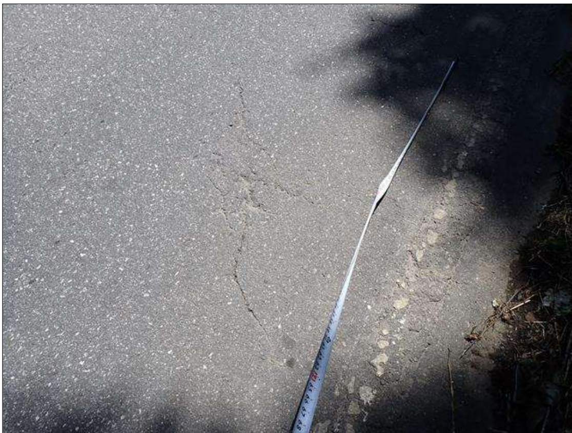
Span 1 Wearing Surface: MULTIPLE AREAS OF BROKEN ASPHALT/MAF CRACKING UP TO 1/16 INCH X 2 FOOT X 10 FOOT SOUTHBOUND LANE 7 FOOT FROM WEST CURB
