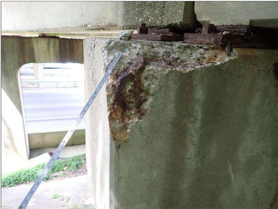
Bent 1 Cap 1: (PAR) 2 FOOT X UP TO 16 INCH X 3 INCH DEEP SPALL WITH EXPOSED RUSTED PRIMARY REINFORCING [SECTION LOSS UP TO 1/8 INCH] AT SOUTHWEST CORNER
