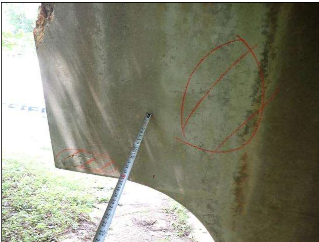
Bent 1 Cap 1: south face, west end, (2) delaminations (up to 13 inch x 19 inch)
