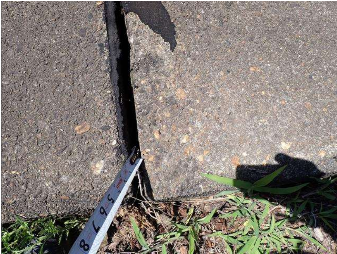
Span 4 Left Bridge Rail: at bent 3 top of curb, spall [3 inch x 11 inch x up to 3/4 inch] no exposed rusted reinforcing
