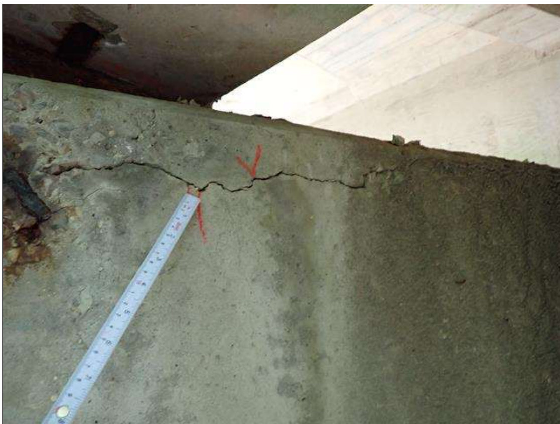
Bent 1 Cap 1: (3) UP TO 3 FOOT X 1/16 INCH HORIZONTAL CRACKS SOUTH AND NORTH FACE BAY 1
