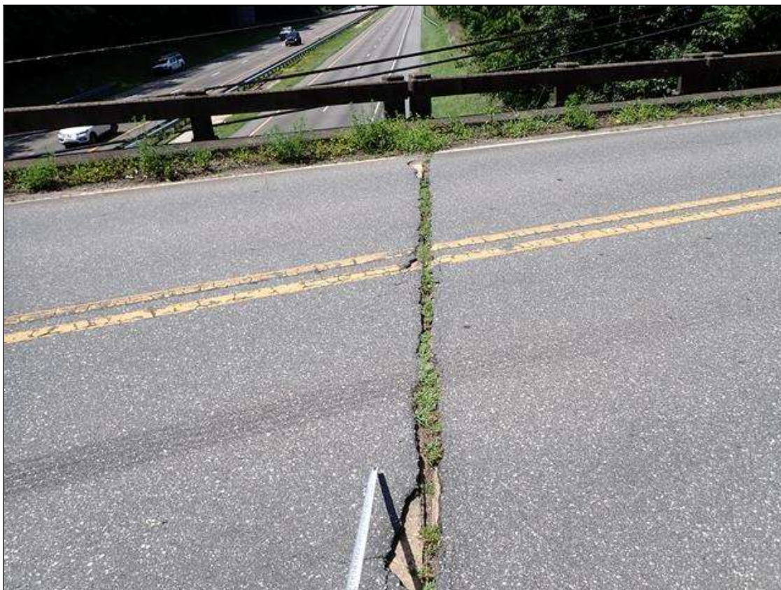
Span 4 Wearing Surface: (PAR) at bent 4, (3) potholes (up to 3 foot x 8 inch x full depth)
