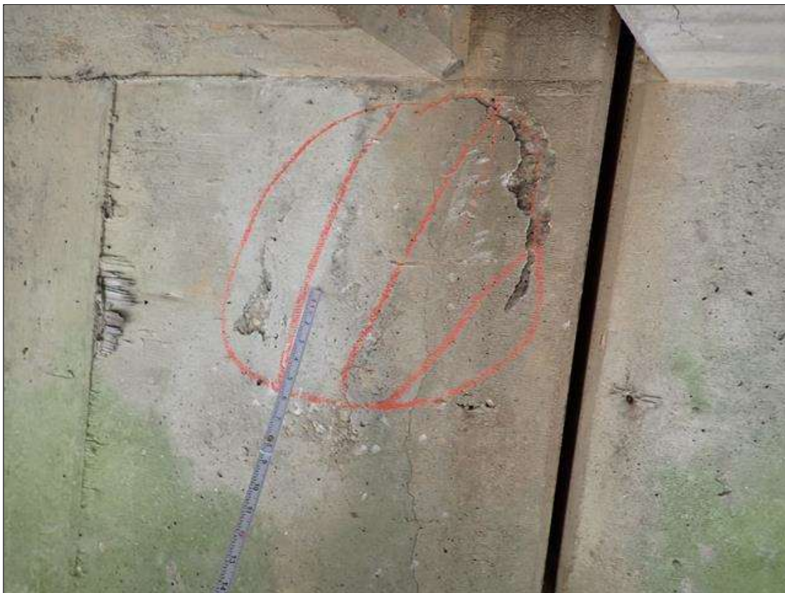
Span 4 Beam 3: west face at bent 3, delamination [16 inch diameter] with cracks [up to 1/32 inch]
