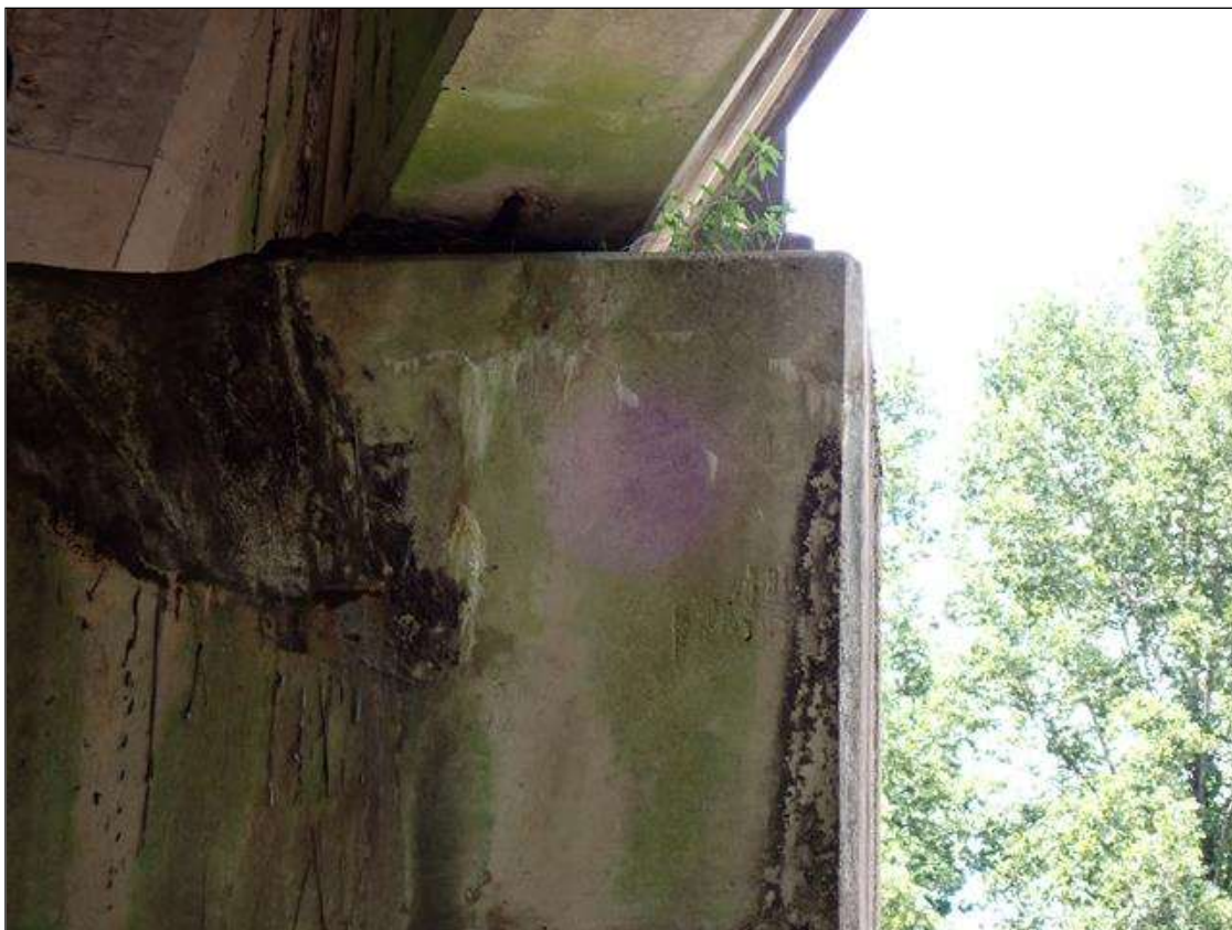
Bent 2 Cap 1: 3 FOOT X UP TO 1/64 INCH HORIZONTAL CRACK WITH EFFLORESCENCE AND ADJACENT 3 FOOT X 8 INCH X 4 INCH DELAMINATION ON TOP SOUTHEAST CORNER
