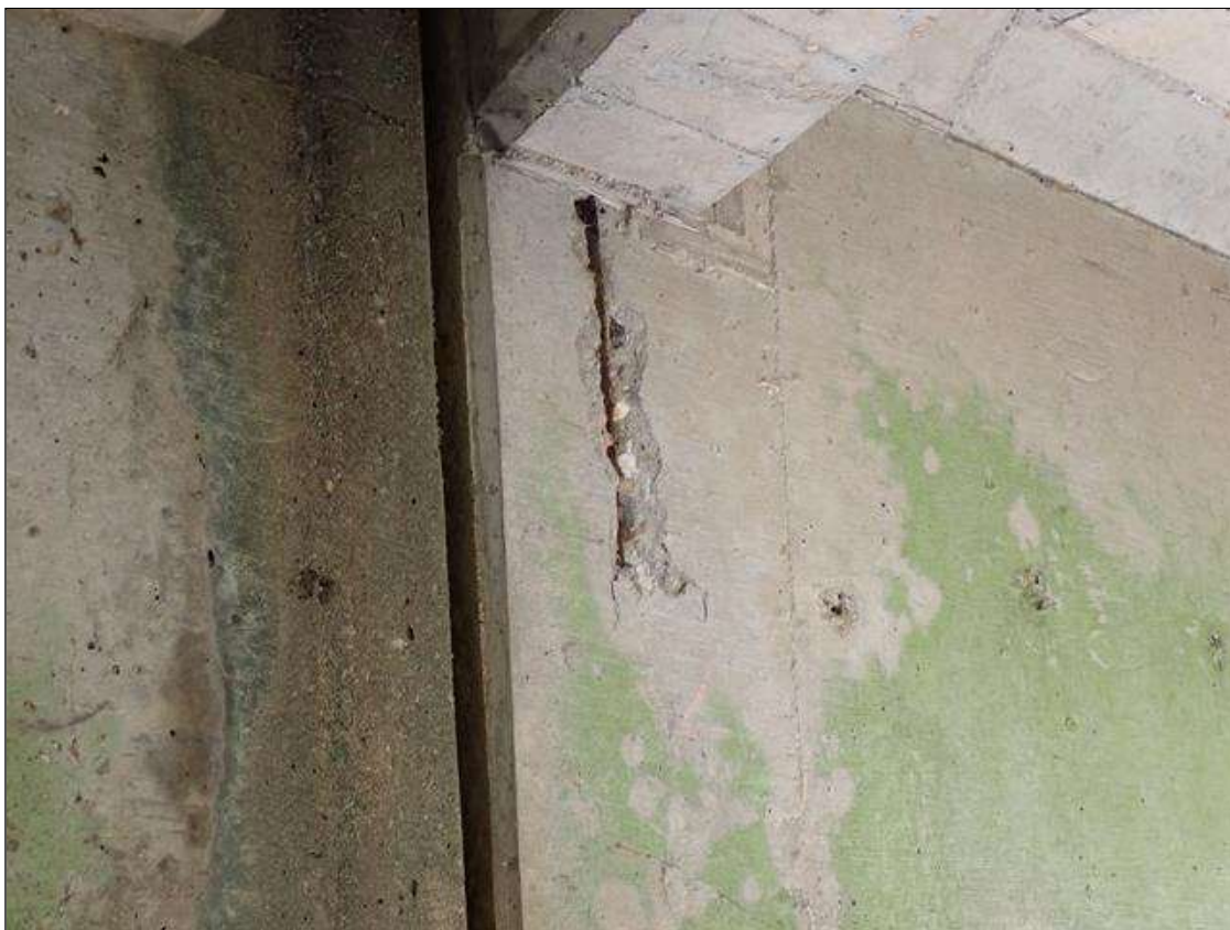
Span 3 Beam 1: east face web at bent 2, spall [12 inch x 2 inch x 1/2inch deep] with exposed rusted reinforcing
