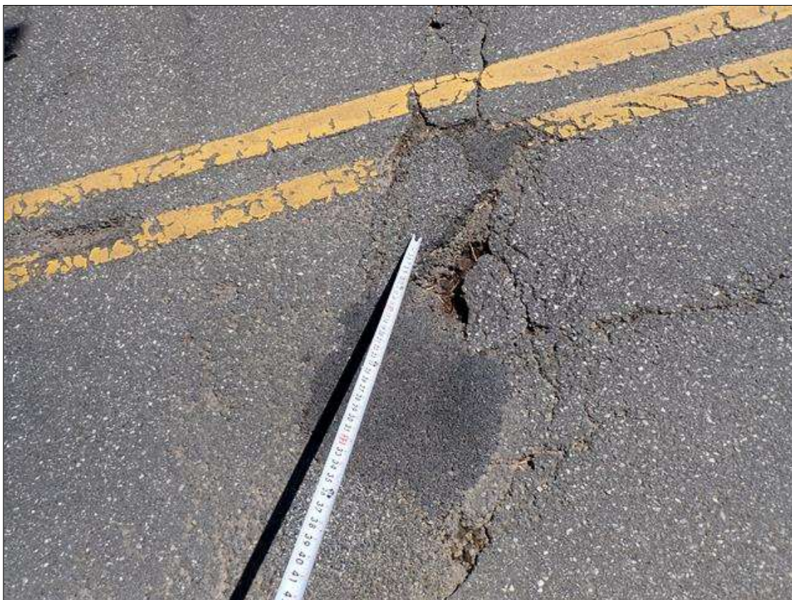
Span 1 Wearing Surface: (PAR) at centerline of roadway, pothole (14 inch x 4 inch x 3 inch deep)
