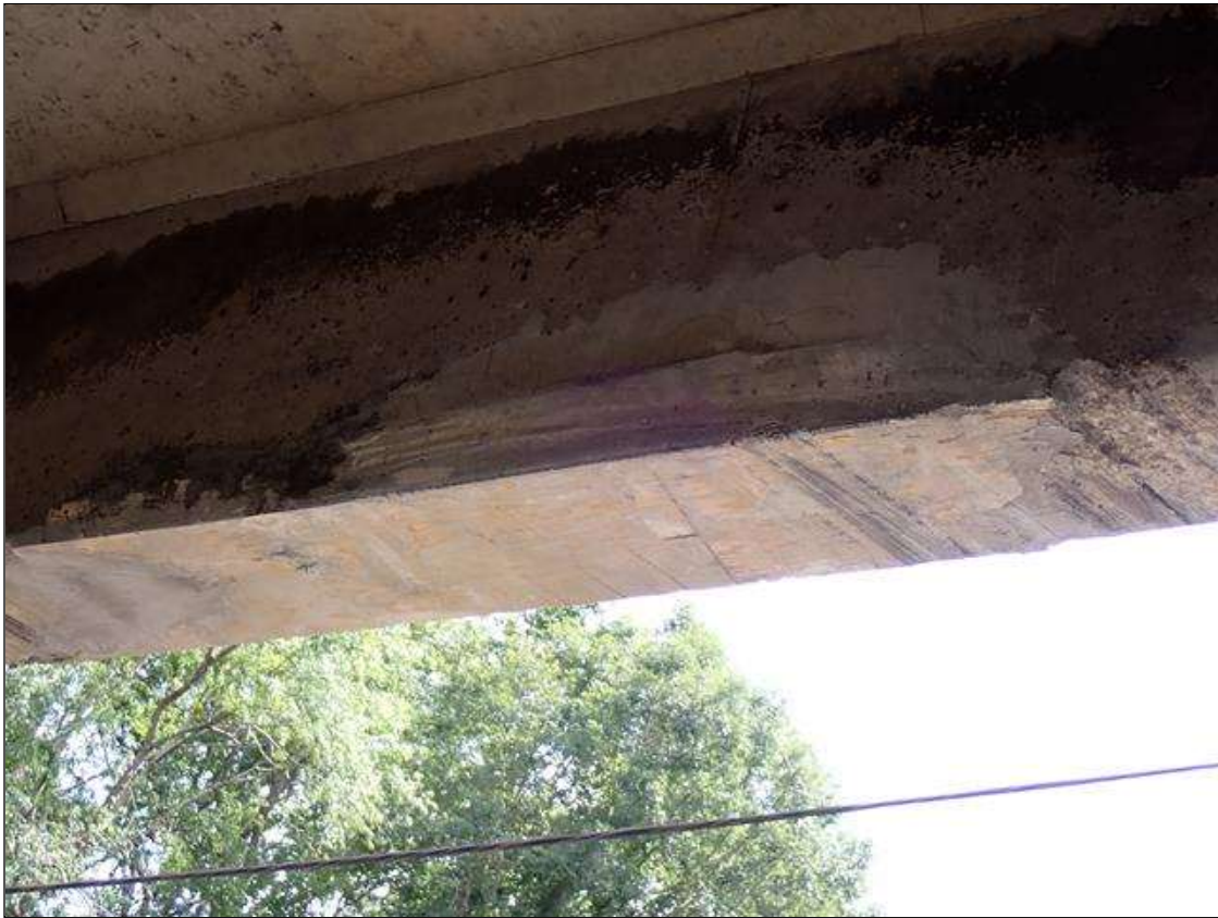
Span 4 Beam 1: 2023 NEW REPAIR, PATCHED AREA, PREVIOUSLY NOTED AS: SUPPLEMENTAL INSPECTION IMPACT DAMAGE 11/23/2021 [PAR] EAST FACE LOWER WEB OVER I-40 RIGHT WESTBOUND LANE, SPALL/IMPACT DAMAGE [14 FOOT X UP TO FULL WIDTH X UP TO 15 INCH UP BOTH FACES X UP TO 3.5 INCH DEEP] WITH MULTIPLE EXPOSED RUSTED PRIMARY REINFORCING [SECTION LOSS UP TO 1/16 INCH] WITH ADJACENT DELAMINATIONS [UP TO 18 INCH X 10 INCH]
