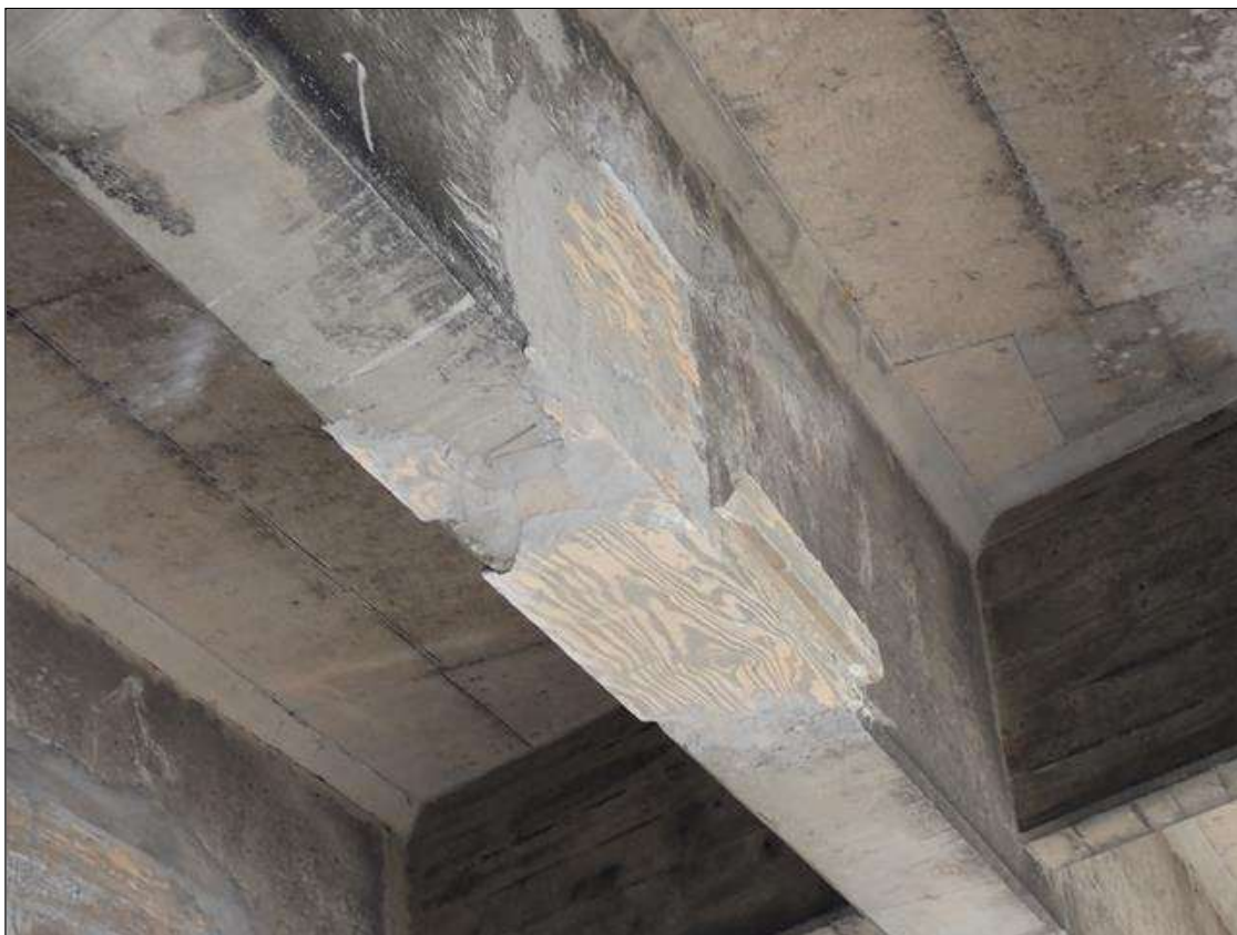
Span 4 Beam 2: 2023 NEW REPAIR, PATCHED AREA, PREVIOUSLY NOTED AS: SUPPLEMENTAL INSPECTION IMPACT DAMAGE 2021 : 2 - UP TO 1.5 FOOT X 10 INCH X 6 INCH SPALLS EAST AND BOTTOM FACE OVER WESTBOUND LANE
