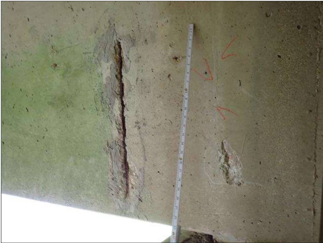
Span 2 Beam 4: at bent 1, west face, (2) delaminations/spalls (up to 3 inch x 2 foot x 1/2 inch deep) with exposed rusted rebar and adjacent cracks (up to 1/32 inch)
