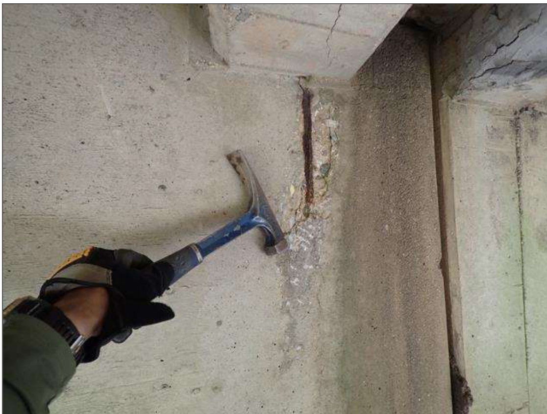
Span 3 Beam 2: east face at bent 3, delamination/spall [3 inch x 1 foot x up to 3/4 inch deep] with exposed rusted reinforcing no section loss
