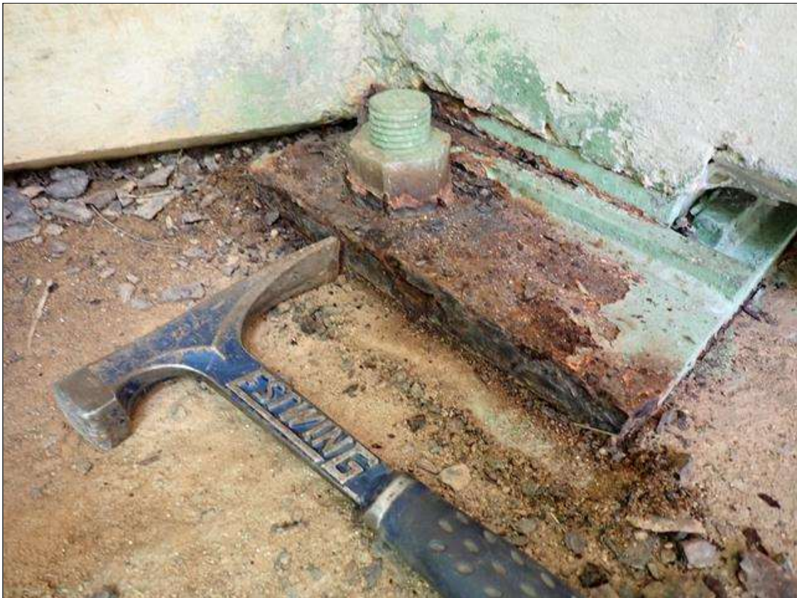
Span 5 Beam 1 - Far Bearing 1: active corrosion with section loss [up to 1/8 inch] on plates
