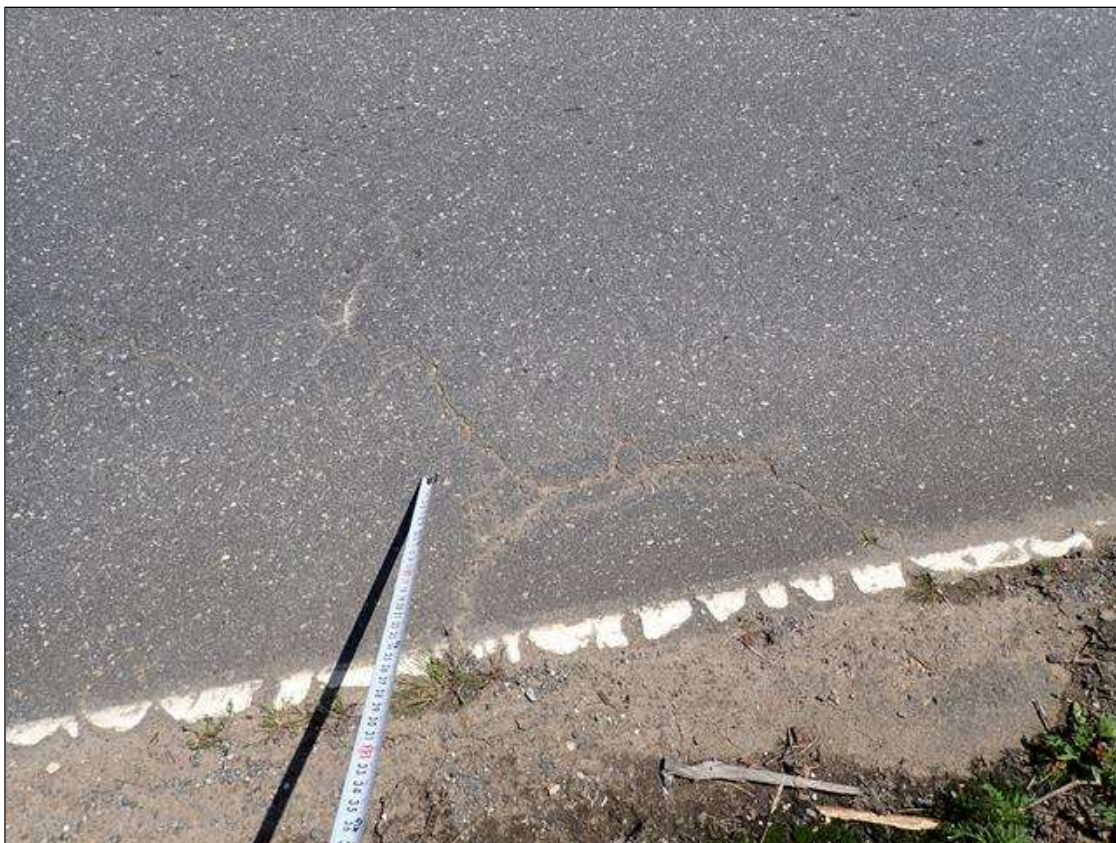
Span 3 Wearing Surface: MAP CRACKING UP TO 1/4 INCH SOUTHBOUND LANE 3 FOOT FROM WEST CURB
