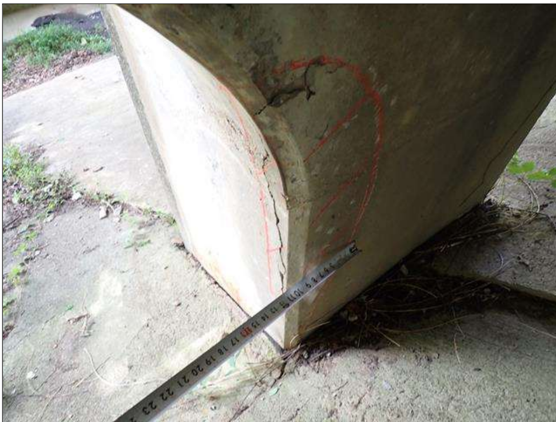
Bent 1 Pile 1: at top of column, southwest corner, delamination (3 foot x 11 inch); southeast corner, vertical crack (up to 1/16 inch x 2 foot)
