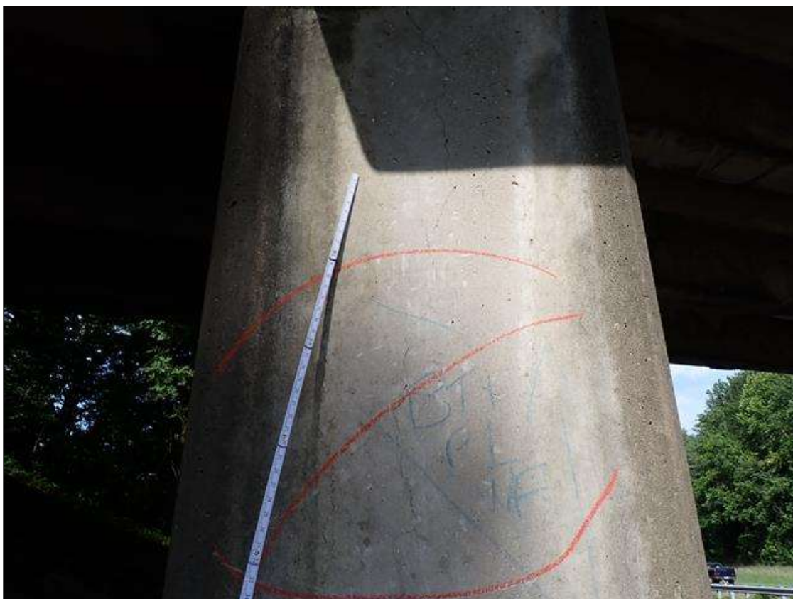
Bent 4 Pile 1: on east and west faces, delamination [up to 4.5 foot x 2 foot] with cracks (up to 1/32 inch)
