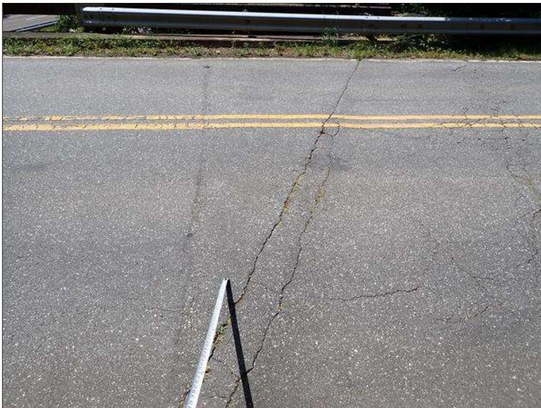
Span 5 Wearing Surface: along length of asphalt over end bent 2, transverse cracks [up to 1/4 inch x full roadway width]
