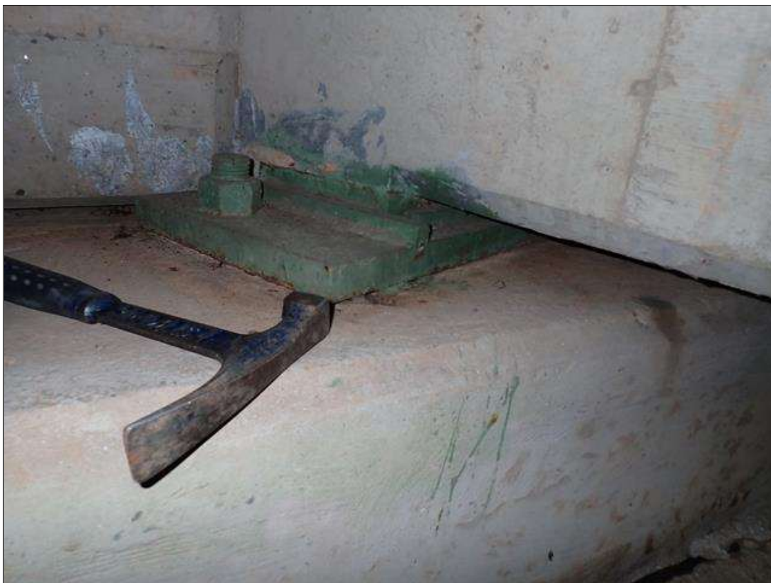
Span 1 Beam 1 - Near Bearing 1: (not found 2023) active corrosion with section loss [up to 1/16 inch] on plates
