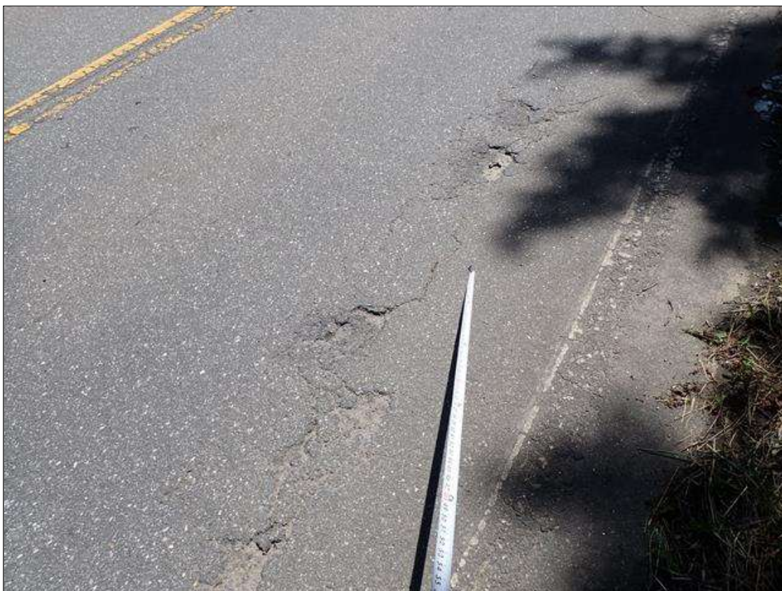
Span 1 Wearing Surface: MULTIPLE AREAS OF BROKEN ASPHALT/MAF CRACKING UP TO 1/16 INCH X 2 FOOT X 10 FOOT SOUTHBOUND LANE 7 FOOT FROM WEST CURB
