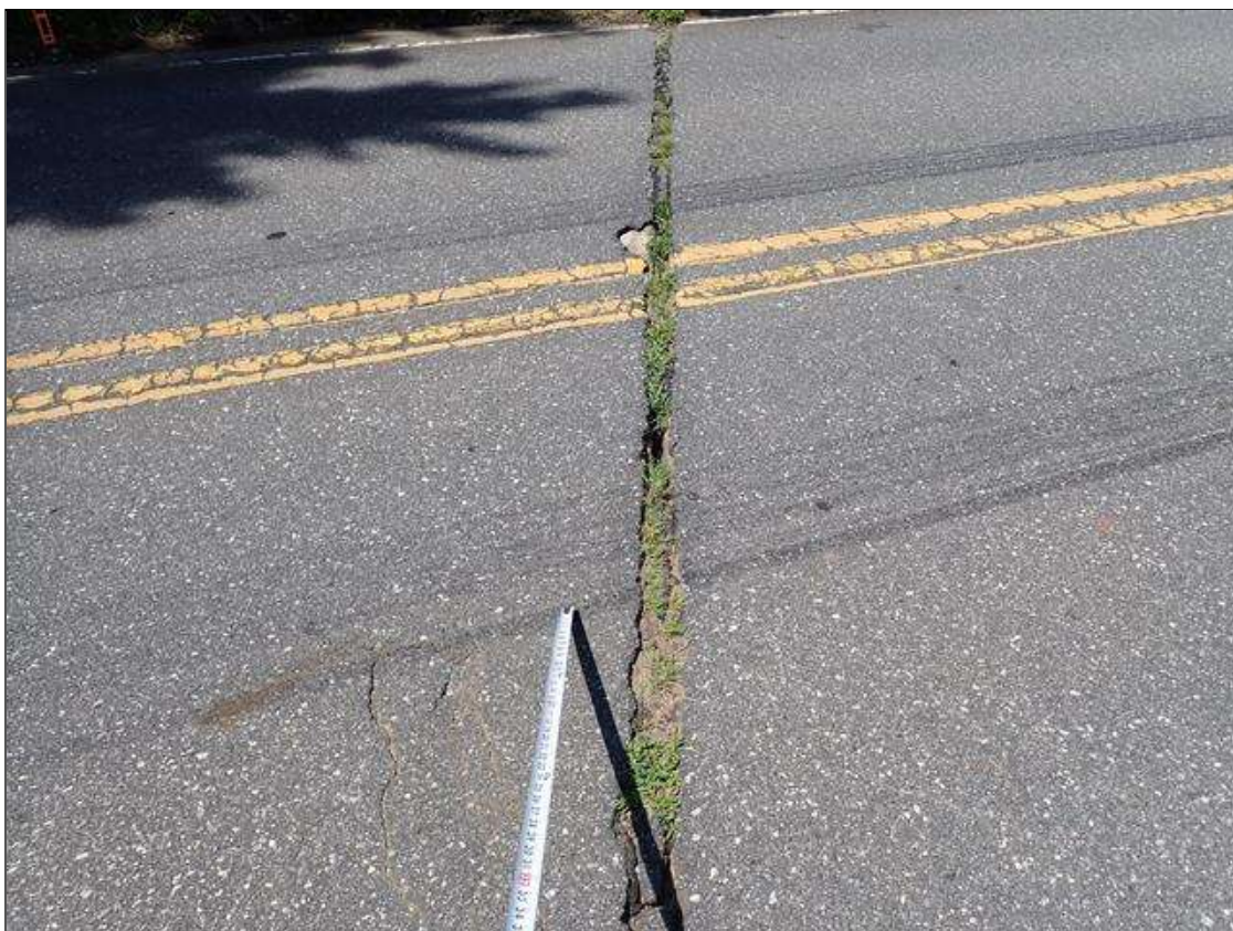
Span 3 Expansion Joint 2: along the length of the joint, joint material deteriorated/torn/missing at random
