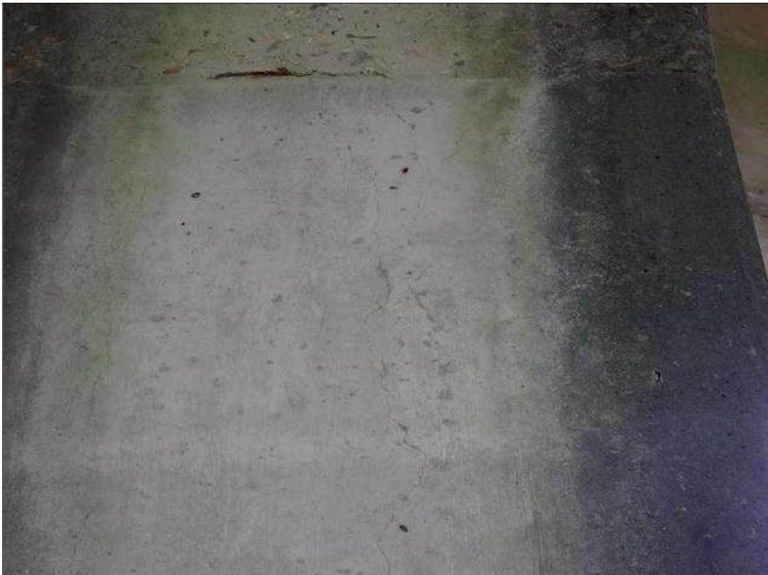
Bent 2 Pile 1: 7 FOOT X UP TO 1/32 INCH VERTICAL CRACKS NEAR BOTTOM OF CAP
