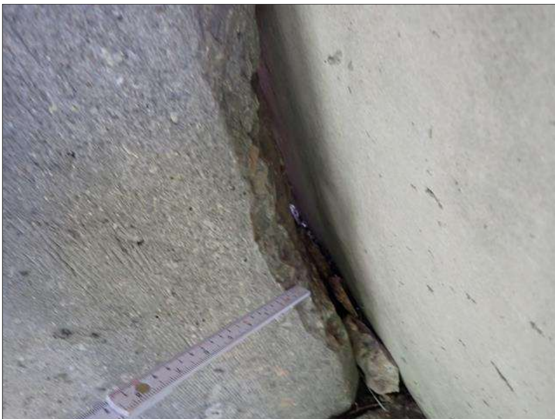
Bent 2 Pile 1: base of column at northeast corner, spall [16 inch x 8 inch x 2 inch deep] with exposed rusted primary reinforcing [no loss noted]
