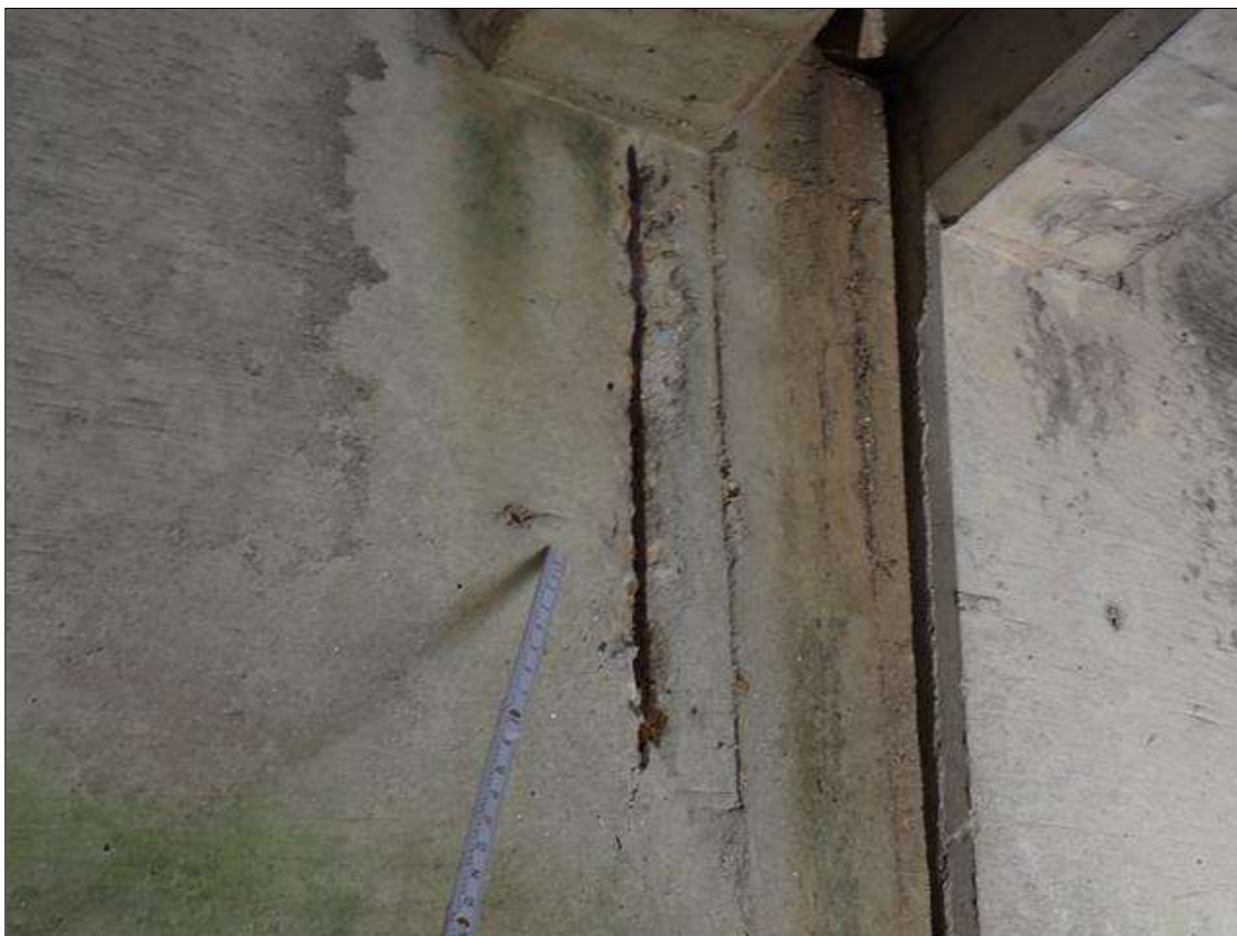
Span 5 Beam 3: west face at bent 4, spall/delamination [2 foot x 3 inch wide x 1/2 inch deep]
