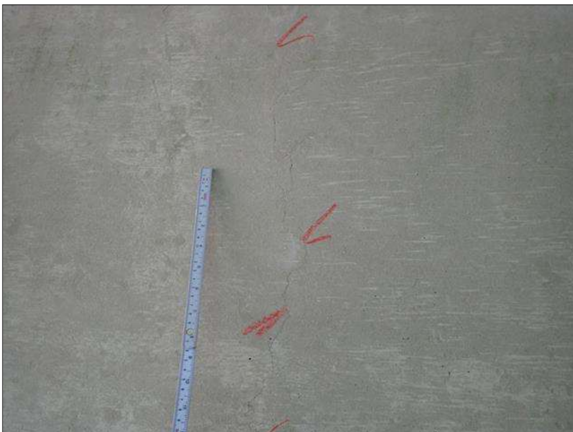
Span 1 Beam 1: TRANSVERSE AND WRAPAROUND CRACKS UP TO 1/64 INCH AT RANDOM THROUGHOUT
