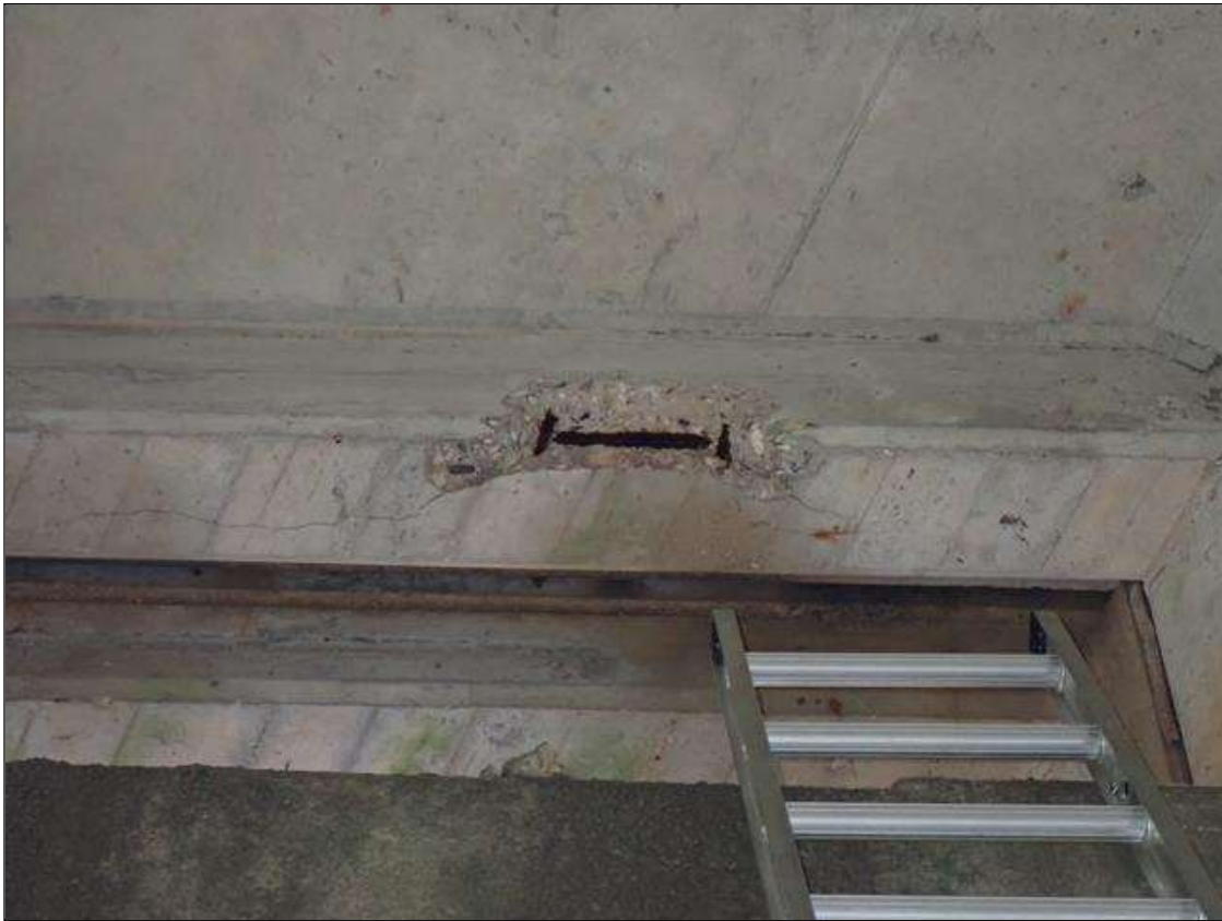
Span 2 Beam 2: at bent 2 bay 2 end diaphragm, spall [22 inch x 3 inch x 3 inch with exposed rusted reinforcing [no loss noted] with cracks [up to 1/16 inch]
