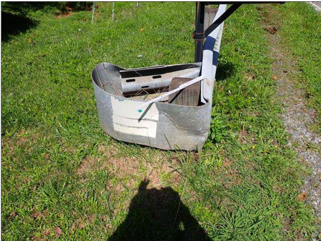
(PAR) southwest guardrail termination, impact damage
