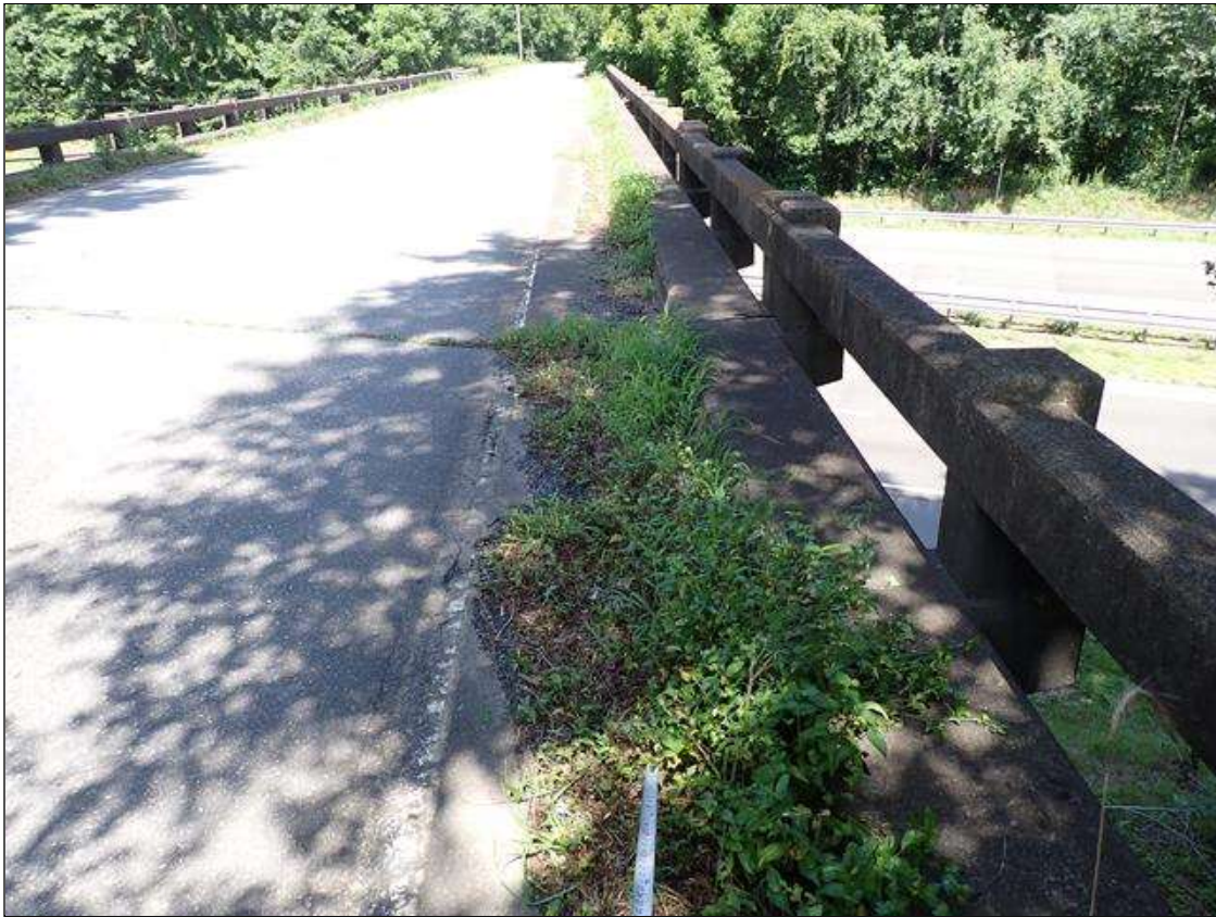
along both curblines, debris accumulation (up to 29 inch x full length) with vegetation growth; fully obstructing deck drainage
