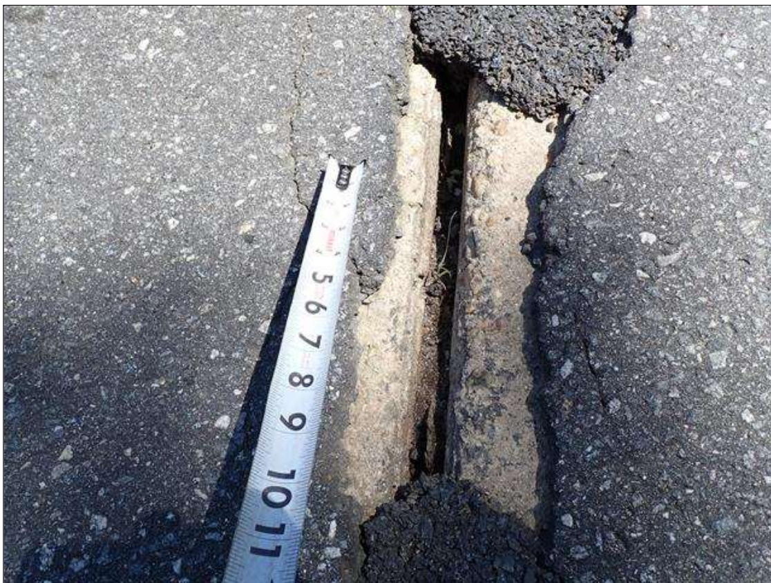
Span 2 Expansion Joint 1: along the length of the joint, joint material deteriorated/torn/missing at random
