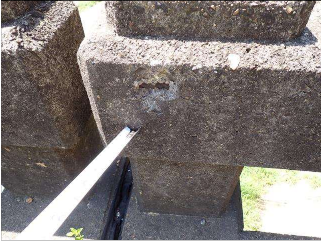
Span 5 Left Bridge Rail: at 1st rail post, spall [3 inch diameter x up to 1 inch deep] with exposed rusted reinforcing [no section loss noted]
