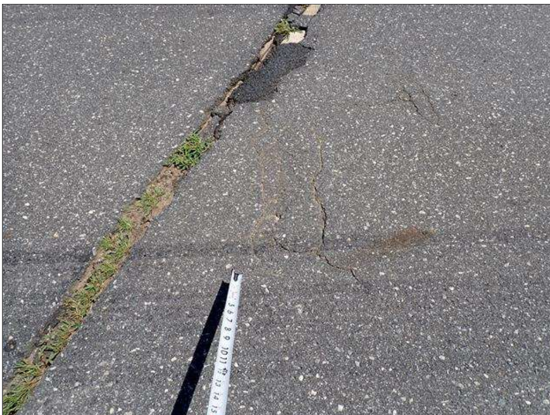
Span 2 Wearing Surface: throughout topside of deck, multiple transverse and longitudinal cracks [up to 16 inch x up to 1/4 inch]
