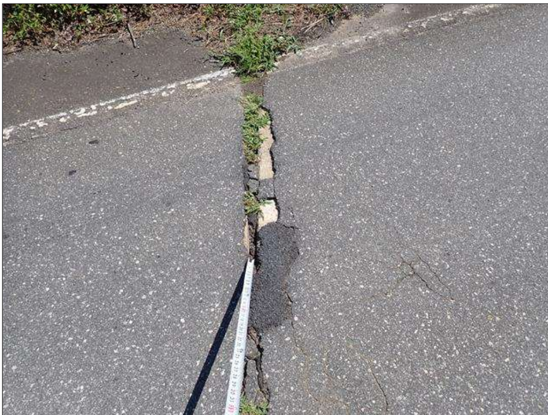
Span 2 Wearing Surface: (PAR) at bent 2, partially patched potholes (up to 16 inch x 6 inch x full depth)
