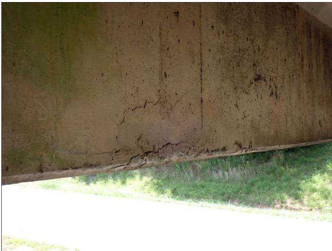
Span 3 Beam 1: (PAR) east face lower web at 5 foot from bent 2, delamination, 5 foot x up to 24 inch high, over right shoulder of I-40 eastbound lane
