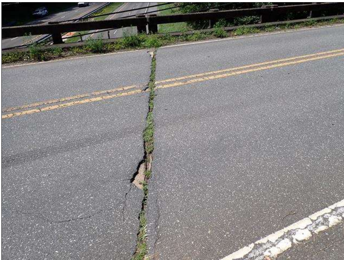
Span 5 Wearing Surface: (not found 2023) 31 INCH X UP TO 1 FOOT X 1 INCH FULL DEPTH POT HOLE OVER BENT 4
