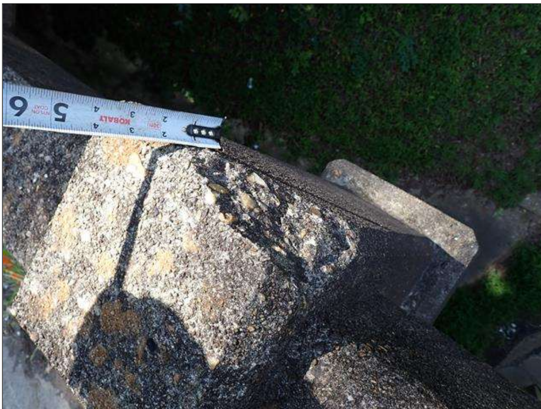
Span 2 Left Bridge Rail: at 5th rail post from bent 1, top corner, spall [4 inch x 3 inch x up to 3/4 inch] no exposed reinforcing
