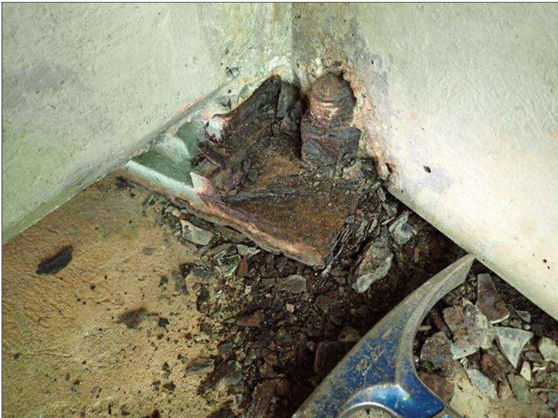
Span 5 Beam 4 - Far Bearing 4: active corrosion with section loss [up to 1/8 inch] on plates
