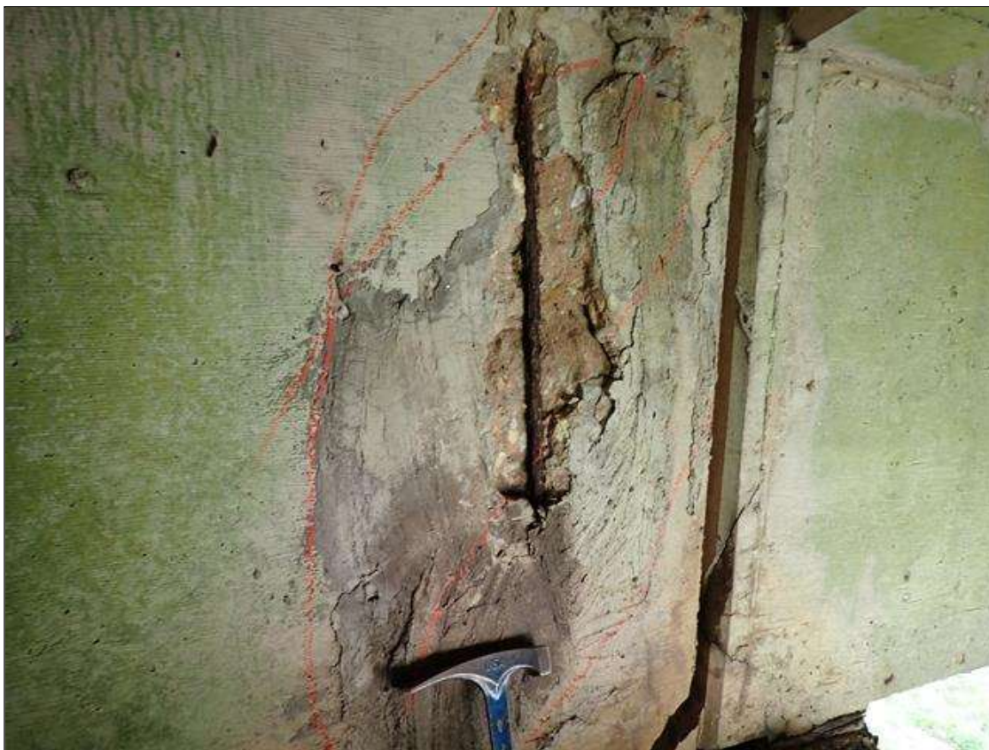
Span 1 Beam 1: (PAR) at bent 1, east face, failed patch (19 inch x full height x 1.5 inch deep) with exposed rusted rebar (approximately 25 percent loss)
