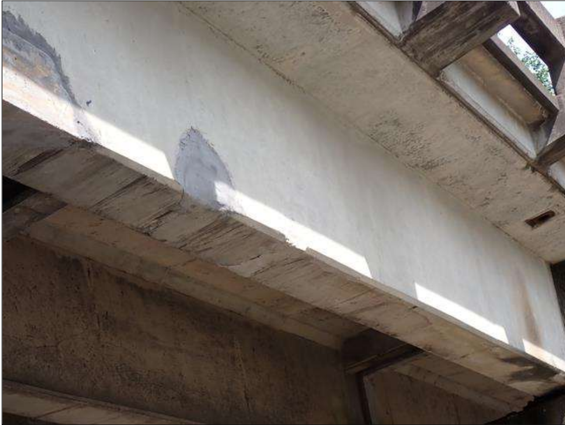
Span 4 Beam 1: 2023 NEW REPAIR, PATCHED AREAS, PREVIOUSLY NOTED AS: SUPPLEMENTAL INSPECTION IMPACT DAMAGE 2021 EAST FACE LOWER WEB OVER I-40 LEFT WESTBOUND LANE, TWO [2] SPALLS/IMPACT DAMAGE [UP TO 14 INCH X FULL WIDTH X 6 INCH] WITH ADJACENT DELAMINATION [UP TO 10 INCH X 8 INCH]
