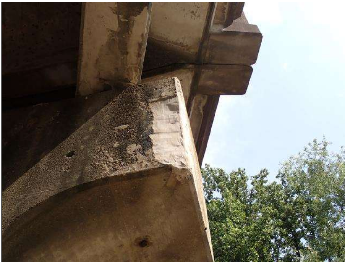
Bent 3 Cap 1: 2023 PREVIOUSLY REPAIRED, PATCHED AREA (3 FOOT X 12 INCH), PREVIOUSLY NOTED AS: 9 INCH X FULL HEIGHT X 10 INCH SPALL WITH EXPOSED RUSTED REINFORCING [SECTION LOSS UP TO 1/16 INCH] NORTH WEST CORNER BENT 3
