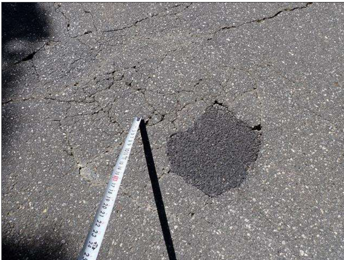
Span 1 Wearing Surface: near end bent 1, northbound lane, patched area (12 inch x 14 inch) with adjacent map cracks (up to 1/16 inch x 2 foot x 2 foot)
