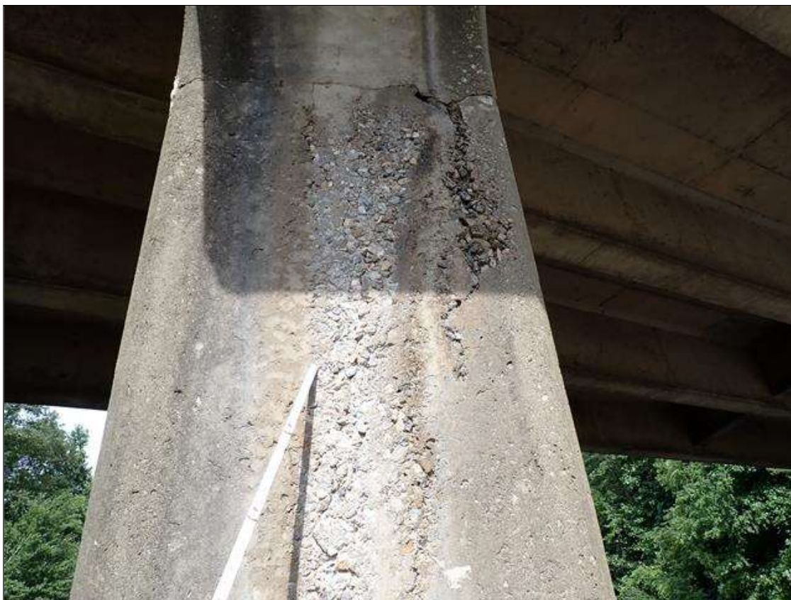
Bent 3 Pile 1: FULL HEIGHT X UP TO 2 FOOT X 1 INCH DEEP AREA OF HONEYCOMBING WEST FACE
