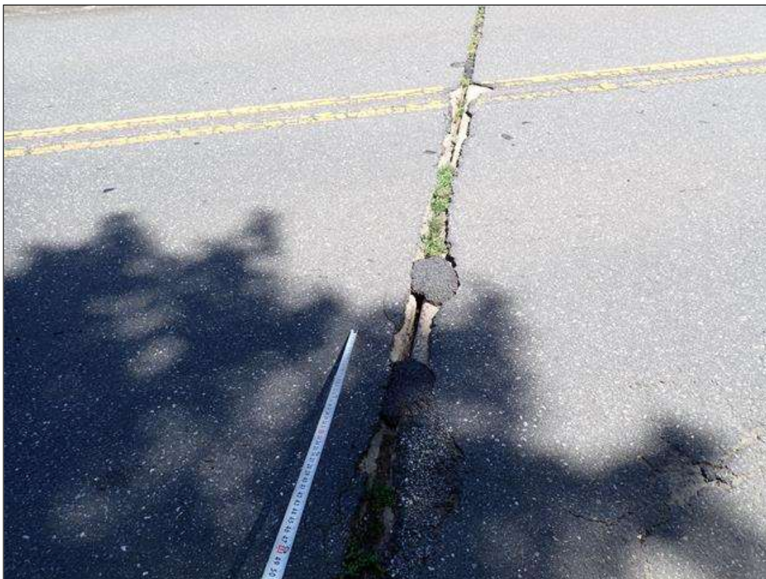
Span 2 Wearing Surface: (PAR) at bent 1, southbound lane, partially patched pothole (13 foot x 6 inch x full depth)
