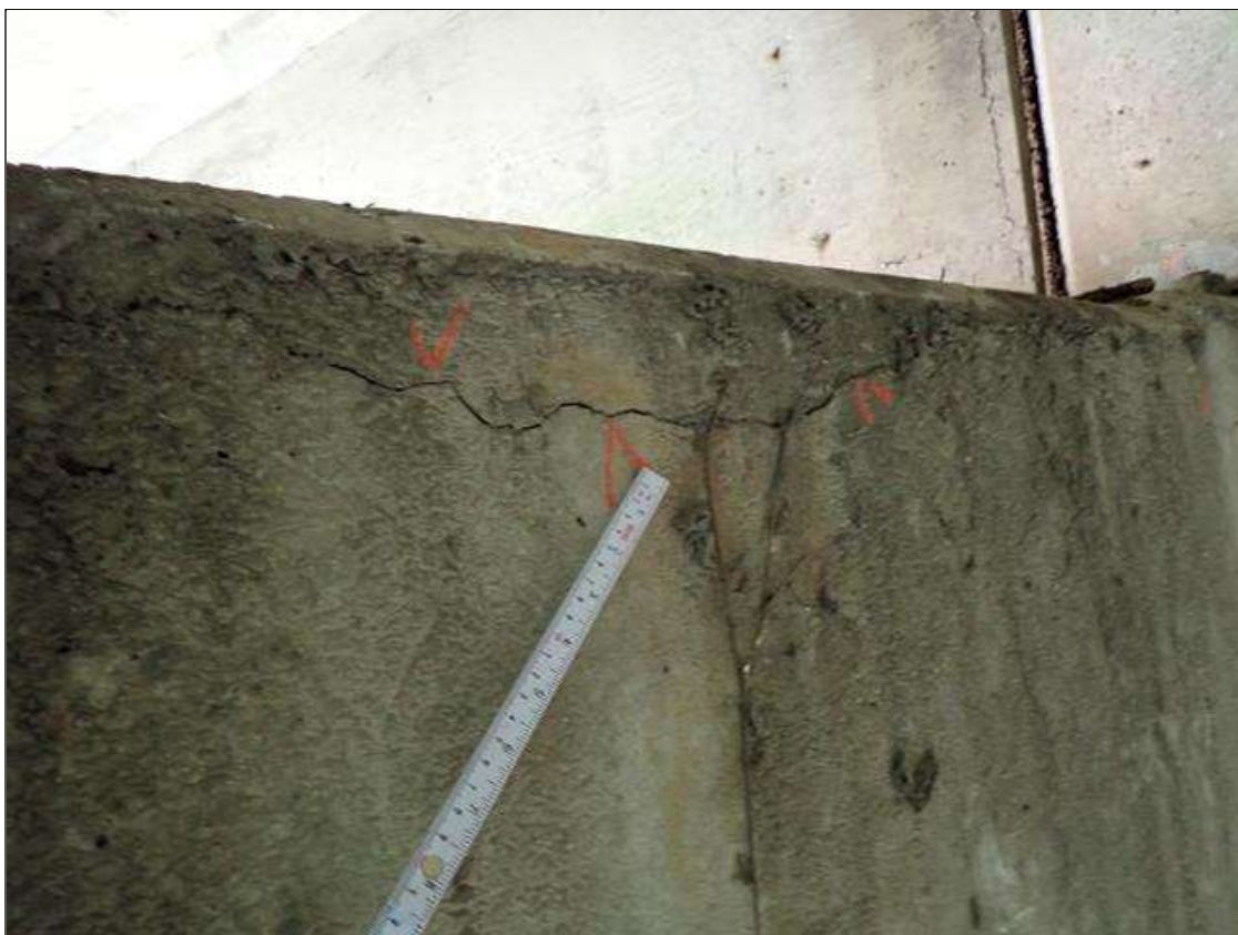
Bent 1 Cap 1: (3) UP TO 3 FOOT X 1/16 INCH HORIZONTAL CRACKS SOUTH AND NORTH FACE BAY 1
