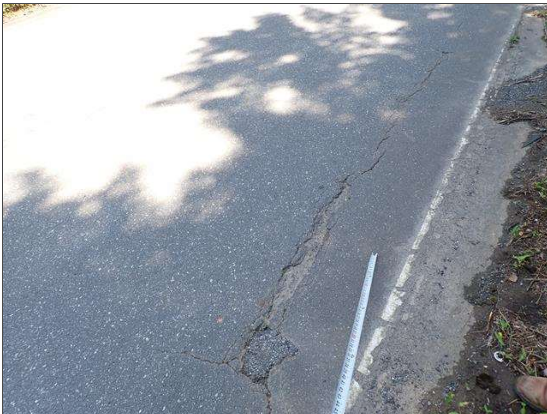
Span 2 Wearing Surface: Southbound lane, shallow pothole/patched area [12 foot long x up to 10 inch x up to 1/2 inch deep]
