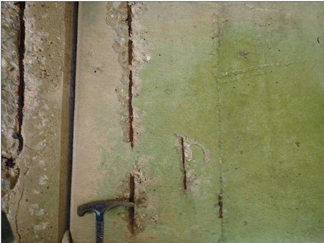
Span 2 Beam 4: (PAR) at bent 2, west face and underside, multiple spalls/delaminations (up to 21 inch x 5 inch x 1 inch deep) with exposed rusted rebar (approximately 25 percent loss)
