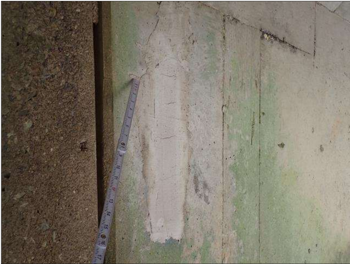
Span 4 Beam 3: 2023 PREVIOUSLY REPAIRED, PATCHED AREA (7 INCH X 2 FOOT) WITH CRACKS (UP TO 1/32 INCH),(PREVIOUSLY NOTED AS: EAST FACE AT BENT 3, DELAMINATION/SPALL [5 INCH X UP TO 4 FOOT X 3/4 INCH DEEP] WITH EXPOSED RUSTED REINFORCING NO SECTION LOSS
