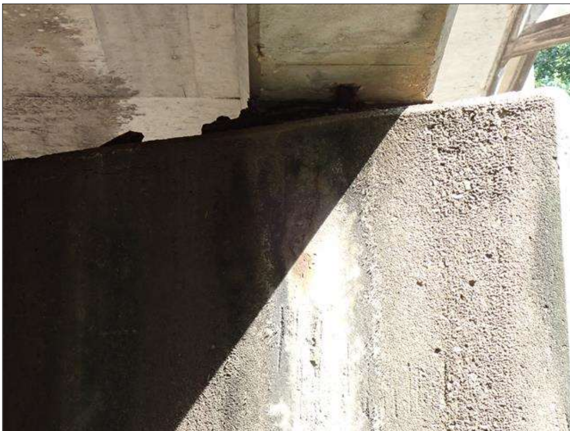
Bent 4 Cap 1: (PAR) 16 INCH X UP TO 1/32 INCH VERTICAL CRACK WITH RUST STAIN NORTH FACE UNDER BEAM 1
