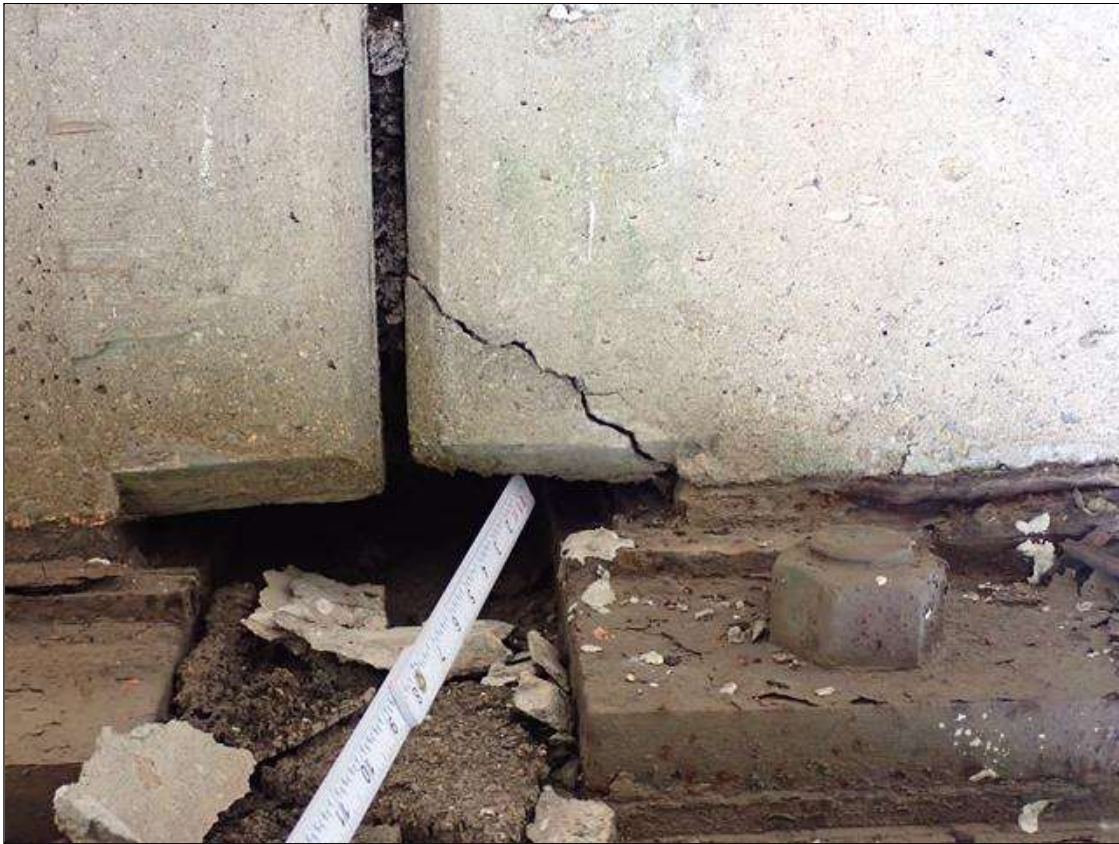
Span 3 Beam 2: at bottom of beam west face at bent 3, delamination (5 inch x 4 inch) with cracks (up to 1/16 inch)
