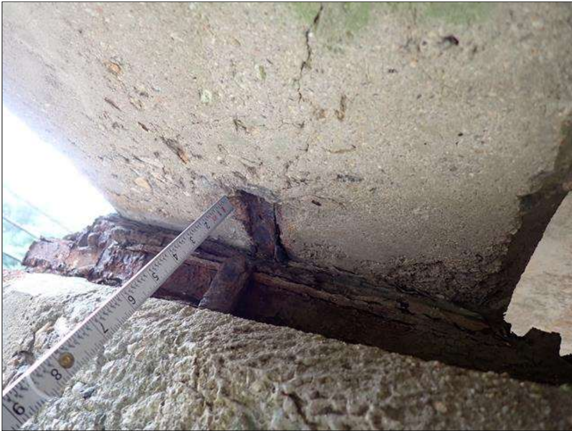
Span 3 Beam 1: at bent 3, east face, spall/delamination (8 inch x 12 inch x 1/2 inch deep); underside, spall (4 inch x 3 inch x 1/2 inch deep) with exposed rusted rebar
