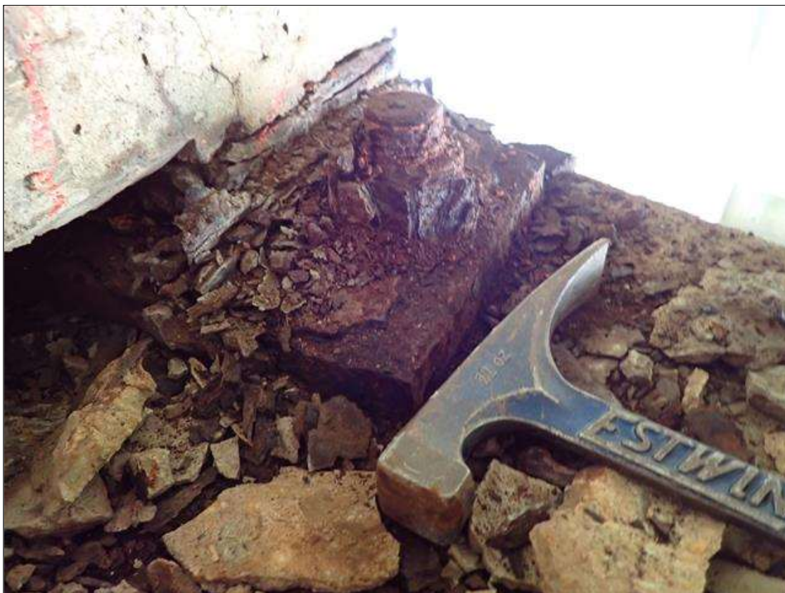
Span 2 Beam 1 - Near Bearing 1: corrosion with section loss (up to 1/8 inch)
