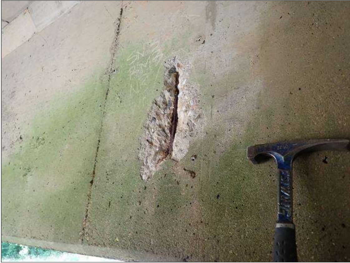
Span 3 Beam 3: west face at bent 2, spall [14 inch x up to 8 inch x 1 inch deep] with exposed rusted reinforcing [no loss noted]; underside at bent 2 bearing, spall [4 inch x 4 inch x 1/2 inch deep] with exposed rusted reinforcing [no loss noted]
