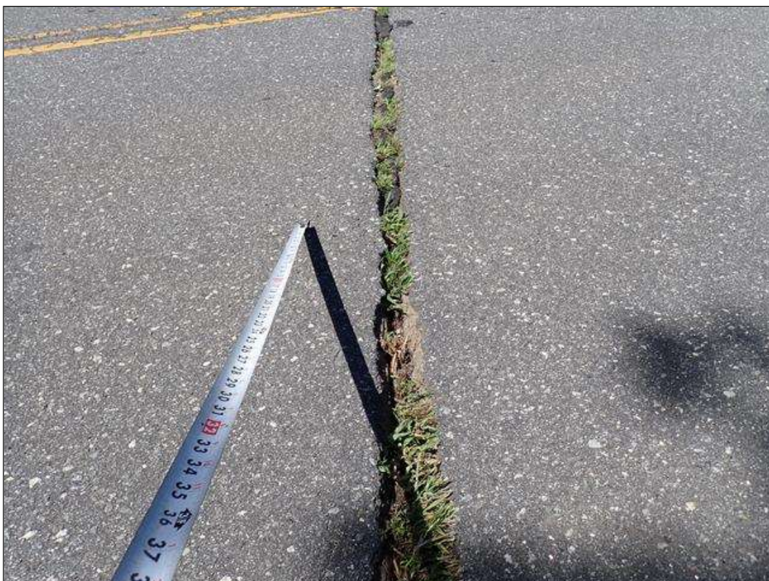
Span 2 Expansion Joint 1: along the length of the joint, joint material deteriorated/torn/missing at random
