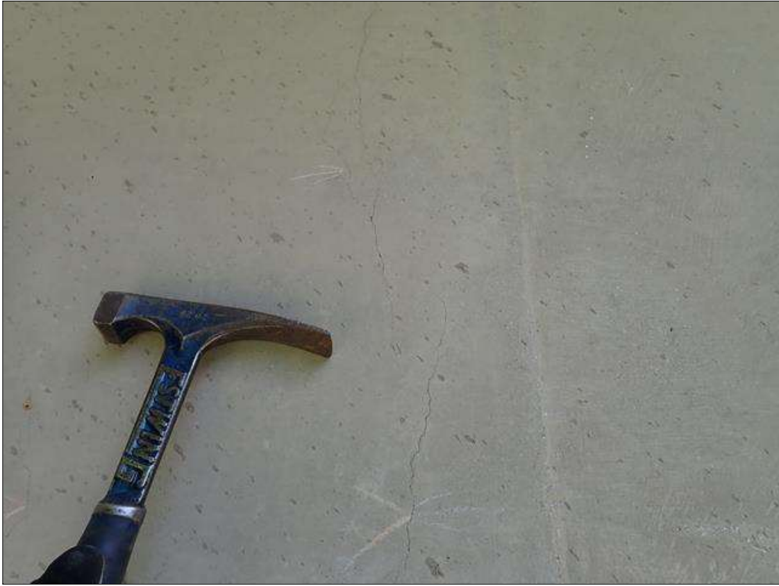
Span 5 Beam 1: VERTICAL CRACKS AND TRANSVERSE AND WRAPAROUND CRACKS UP TO 1/32 INCH AT RANDOM THROUGHOUT
