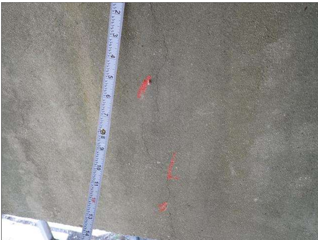
Bent 3 Cap 1: along the length of the cap, vertical cracks (up to 1/64 inch x full height) and longitudinal cracks (up to 1/32 inch x 6 foot) at random
