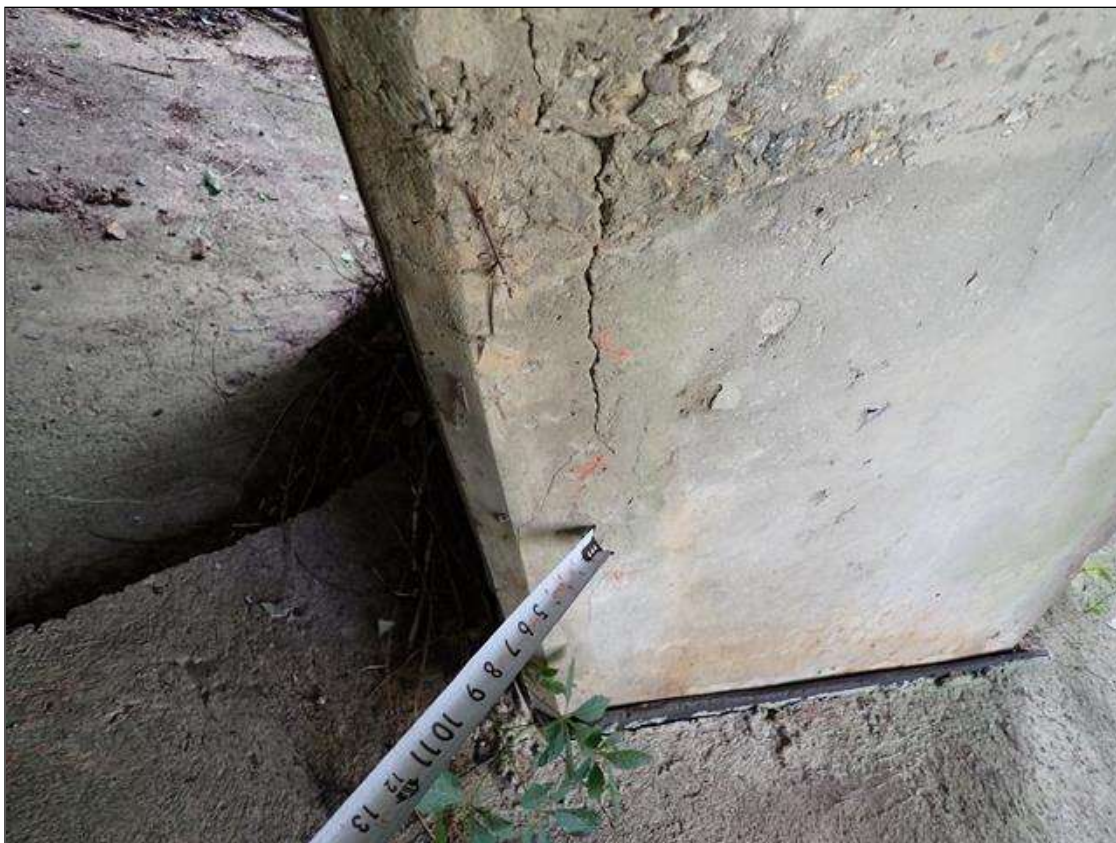
Bent 1 Pile 1: at top of column, southwest corner, delamination (3 foot x 11 inch); southeast corner, vertical crack (up to 1/16 inch x 2 foot)
