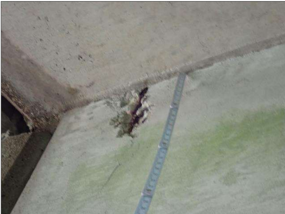
Span 1 Beam 1: West face at bent 1, spall/delamination [12 inch x 3 inch x 1 inch deep] with exposed rusted rebar
