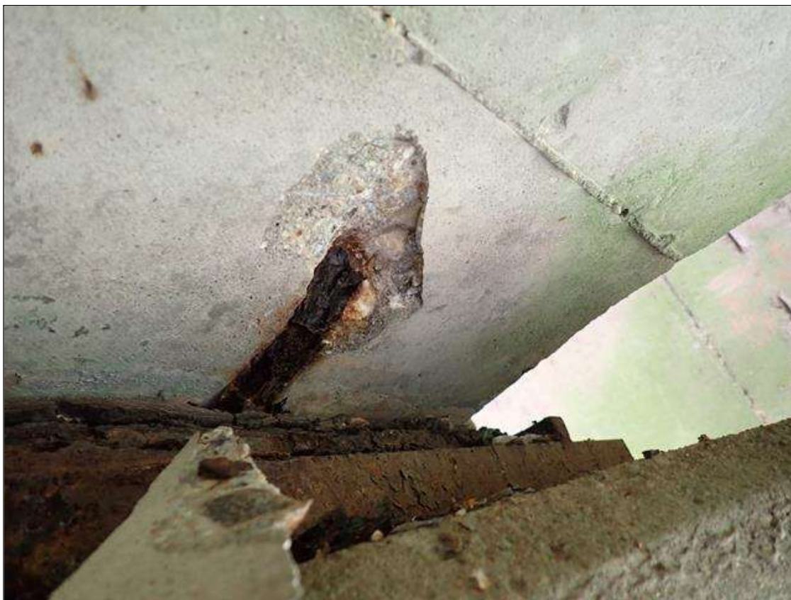
Span 2 Beam 3: at bent 2, underside, spall (6 inch x 3 inch x 1/2 inch deep) with exposed rusted rebar
