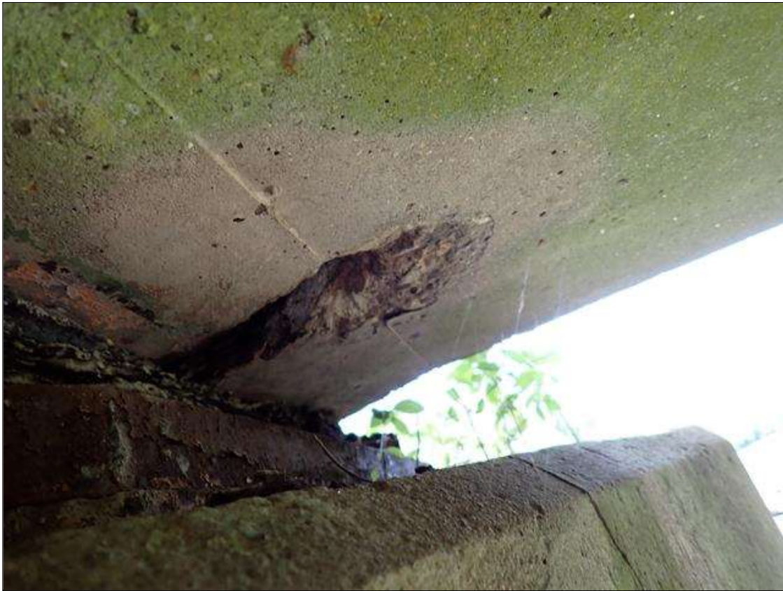
Span 2 Beam 4: (PAR) at bent 2, west face and underside, multiple spalls/delaminations (up to 21 inch x 5 inch x 1 inch deep) with exposed rusted rebar (approximately 25 percent loss)
