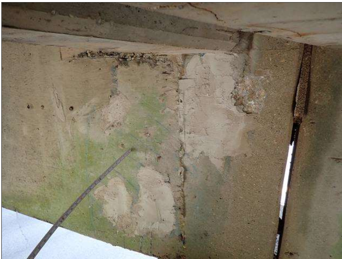
Span 4 Beam 4: 2023 previously repaired, partially sound patches (up to 17 inch x 11 inch x 1 inch deep), previously noted as: West face at bent 3, delamination/spall [4.5 foot x 2 foot x 1.25 inch deep] with (3) exposed rusted reinforcing [section loss up to 1/32 inch]
