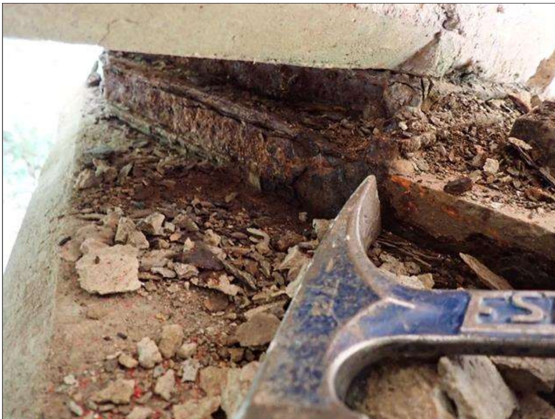
Span 1 Beam 1 - Far Bearing 1: active corrosion with section loss [up to 1/8 inch] on plates
