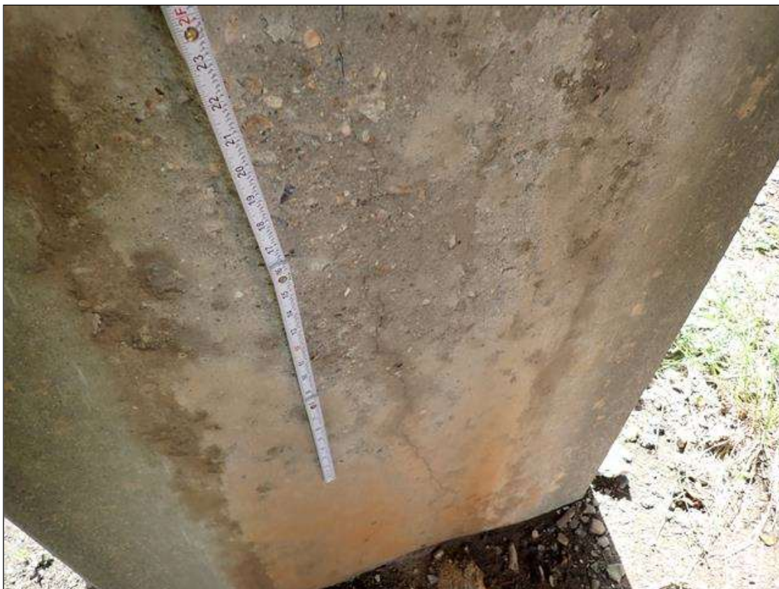
Bent 3 Pile 1: along length of the column, vertical cracks (up to 1/32 inch x full height) at random
