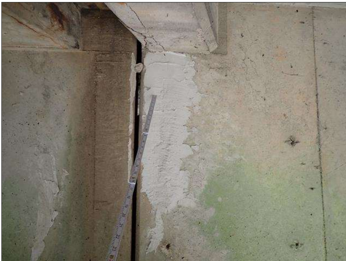
Span 3 Beam 2: 2023 previously repaired, patch (7 inch x 2 foot), previously noted as: West face at bent 3, delamination/spall [5 inch x 3 foot high x up to 3/4 inch deep] with exposed rusted reinforcing no section loss
