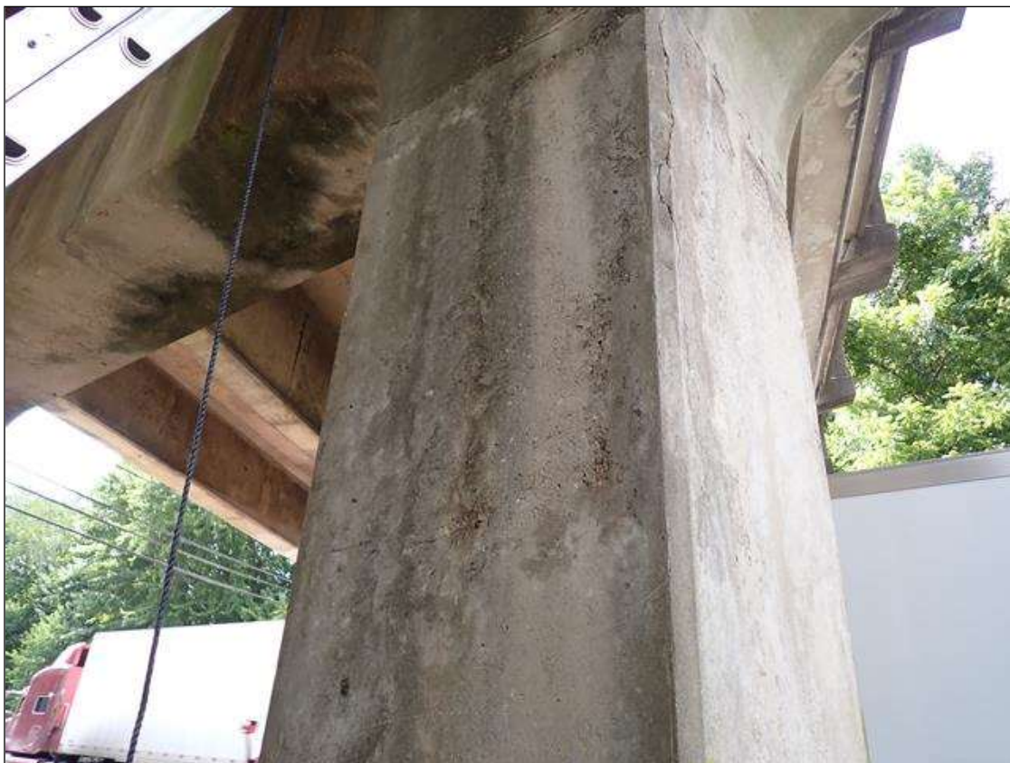
Bent 3 Pile 2: (not found 2023) South face of pile, delamination [2 foot x 6 foot]
