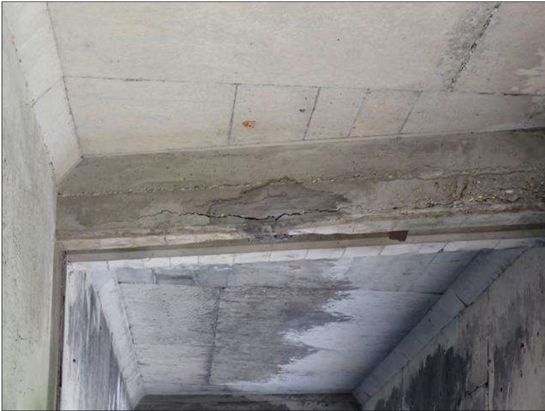
Span 5 Beam 1: span 5 bay 1 near diaphragm failed patch with crack (up to 1/4 inch x full width)
