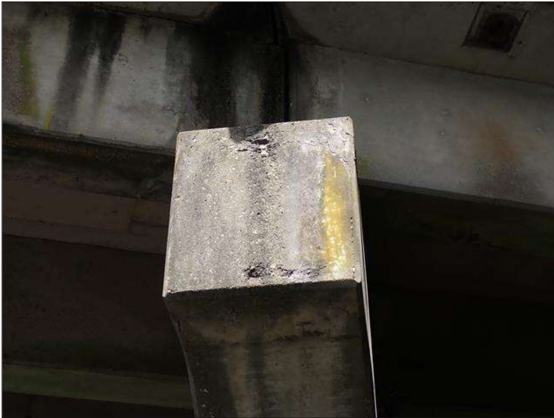
Bent 2 Cap 1: WEST END. HAS SCATTERED AREAS THAT ARE CRACKED UP TO 1/32 INCH AND DELAMINATED WITH SOME POP-OUTS UP TO 1/2 INCH DEEP
