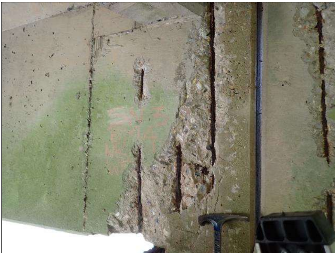
Span 3 Beam 4: (PAR) west face web and underside at bent 2, spall/delamination [30 inch x up to full height x up to 2 inch deep] with exposed rusted primary reinforcing [approximately 25 percent loss]
