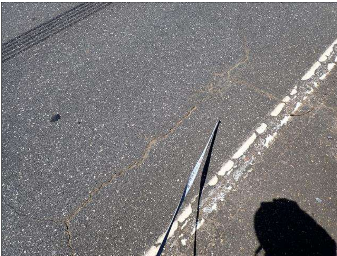
Span 4 Wearing Surface: MAP CRACKING UP TO 1/4 INCH AT RANDOM THROUGHOUT TOPSIDE OF DECK
