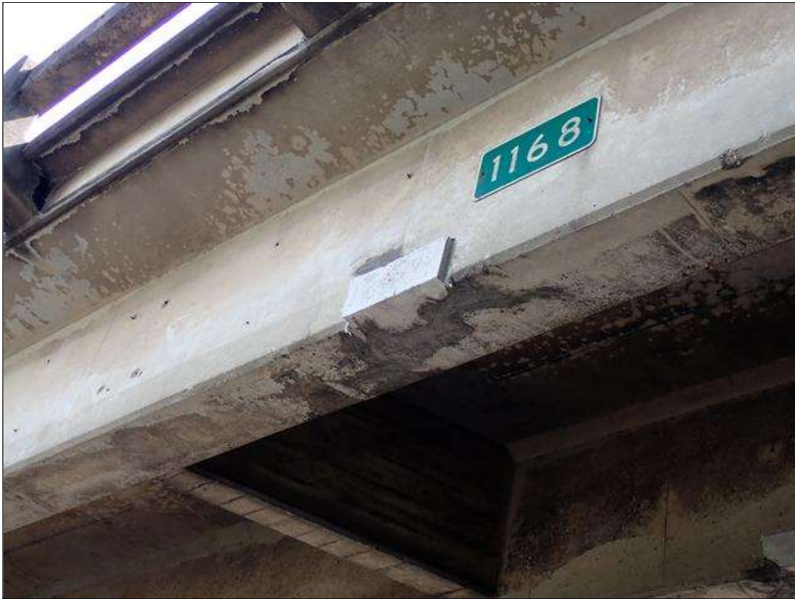
Span 4 Beam 4: 2023 NEW REPAIR, PATCHED AREA, PREVIOUSLY NOTED AS: SUPPLEMENTAL INSPECTION IMPACT DAMAGE 2021 UNDERSIDE OVER I-40 RIGHT WESTBOUND LANE, MULTIPLE SPALLS/AREAS IMPACT DAMAGE [UP TO 3 INCH X 2 INCH X 1/2 INCH DEEP]
