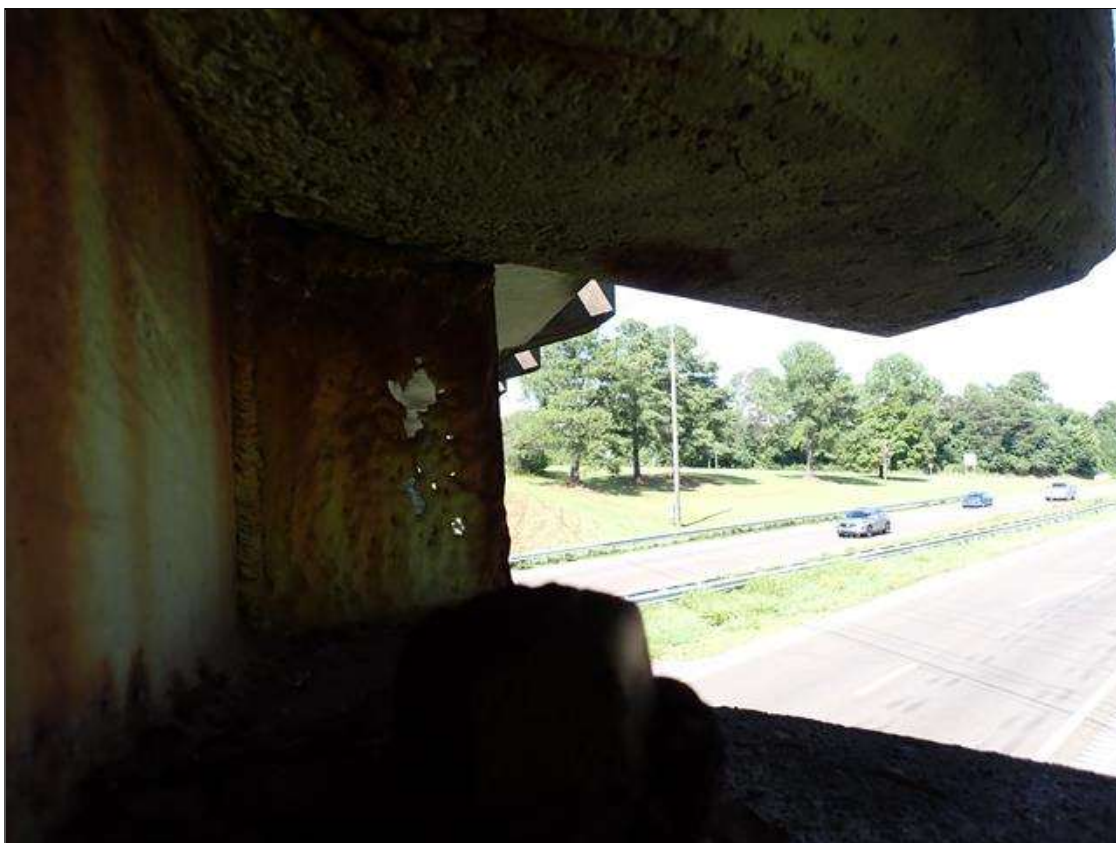
Span 2 Beam 4: (PAR) at bent 1, web adjacent to diaphragm, rust scale (10 inch); right stiffener (0.20 inch average remaining x full width x full height) with corrosion holes (up to 2 inch x 1 inch)
