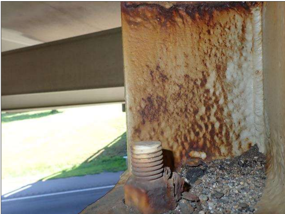
Span 2 Beam 1: at bent 2, corrosion with section loss: web adjacent to diaphragm (1/2 inch average remaining x 10 inch x 1 inch); right stiffener (0.30 average remaining x full width x full height)
