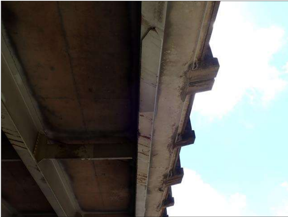
Span 3 Beam 1: underside of coverplate over right travel lane, impact scrapes with surface rust
