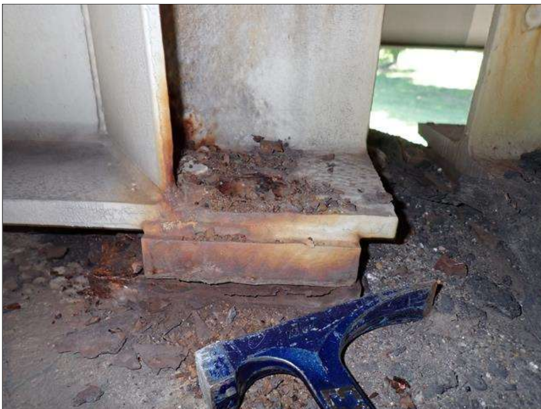
Span 3 Beam 3 - Near Bearing 3: [PAR] right and left attachment bolt sheared
