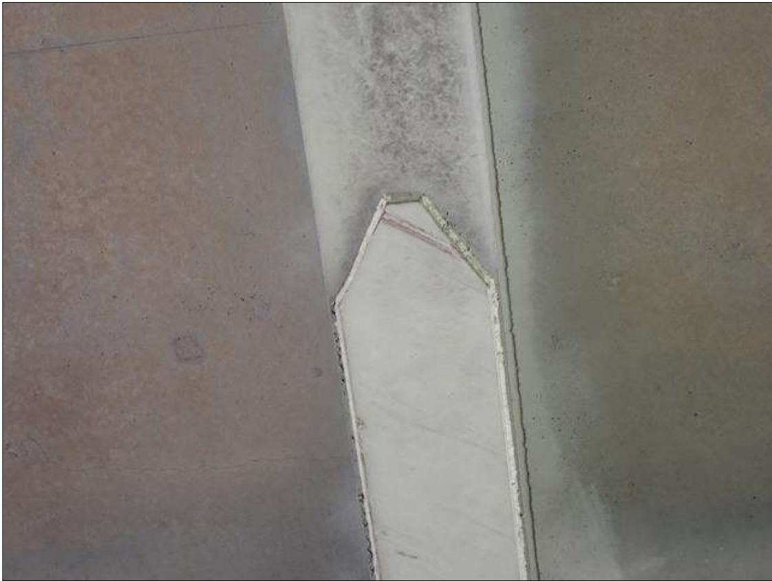
Span 3 Beam 3: underside of coverplate over both travel lanes, impact scrapes with surface rust
