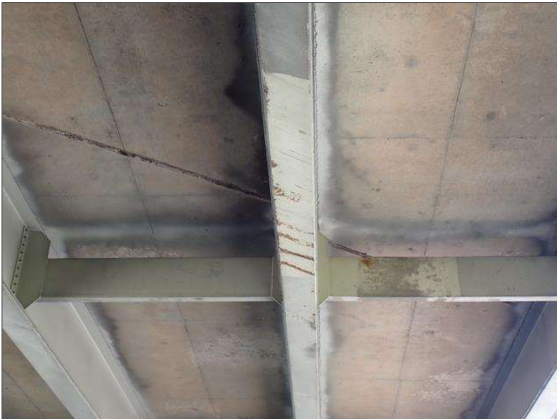
Span 3 Beam 2: underside of coverplate over right travel lane, impact scrapes with surface rust
