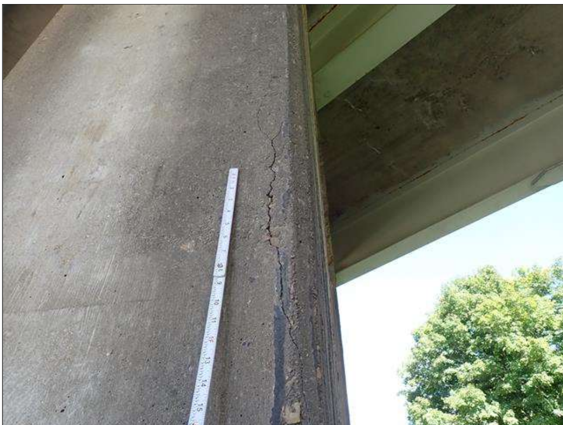
Bent 1 Pile 2: 2.5 FOOT X UP TO 1/16 INCH VERTICAL CRACK ON WEST FACE 6 INCH FROM BOTTOM OF CAP
