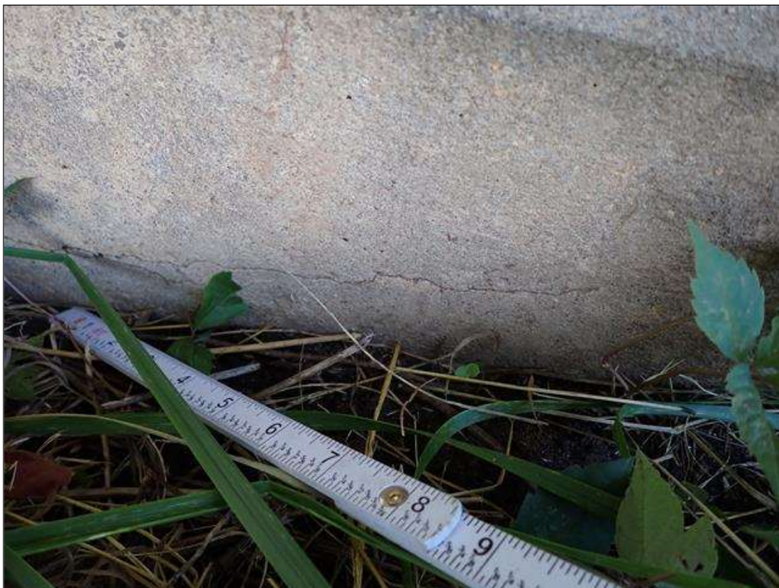
End Bent 2 Cap 1: 16 FOOT X UP TO 1/16 INCH HORIZONTAL CRACK SOUTH FACE BEGINNING AT EAST END
