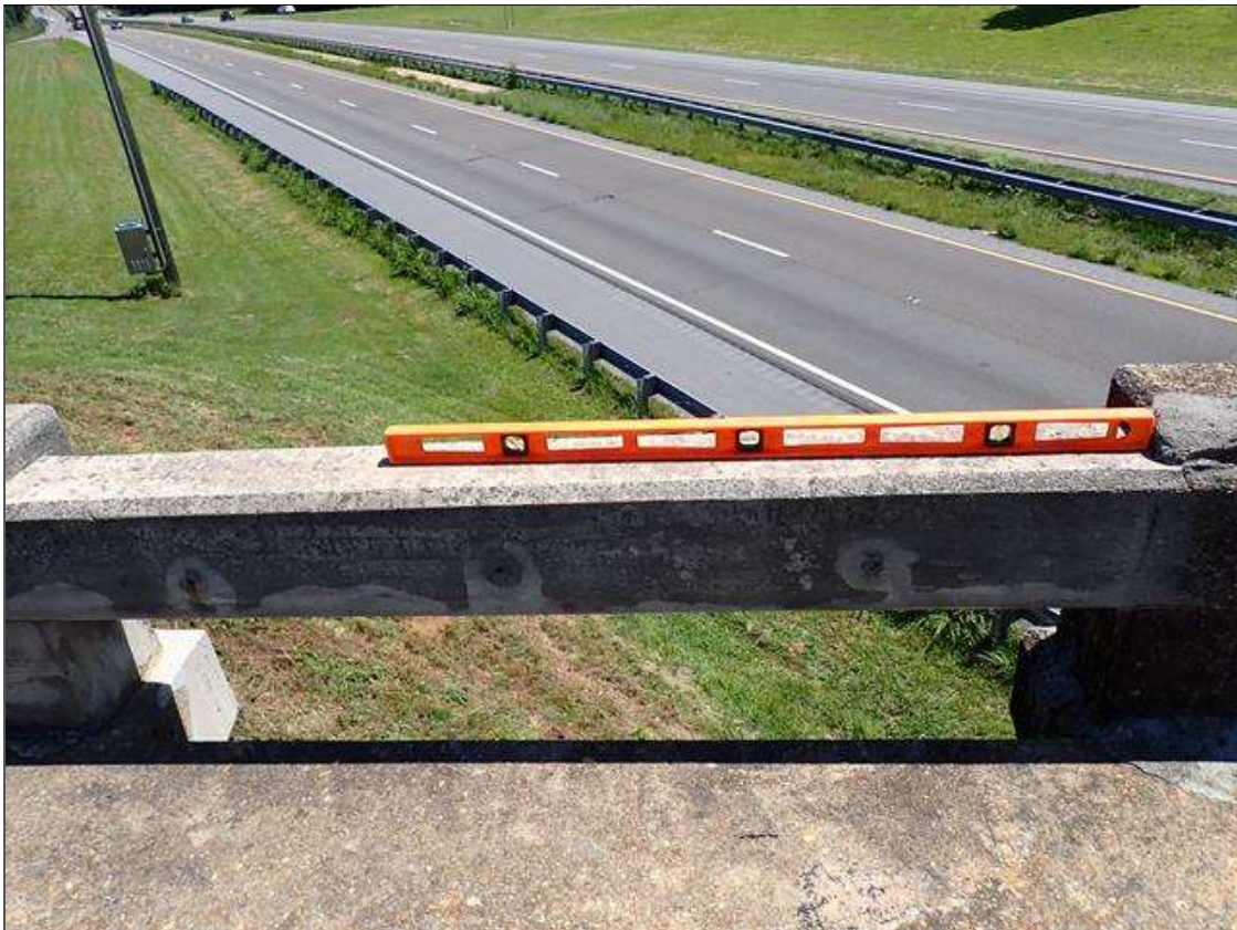
Span 4 Right Bridge Rail: SPAN 4 RIGHT RAIL HAS A REPAIR AREA BETWEEN POSTS 5 AND 6.
