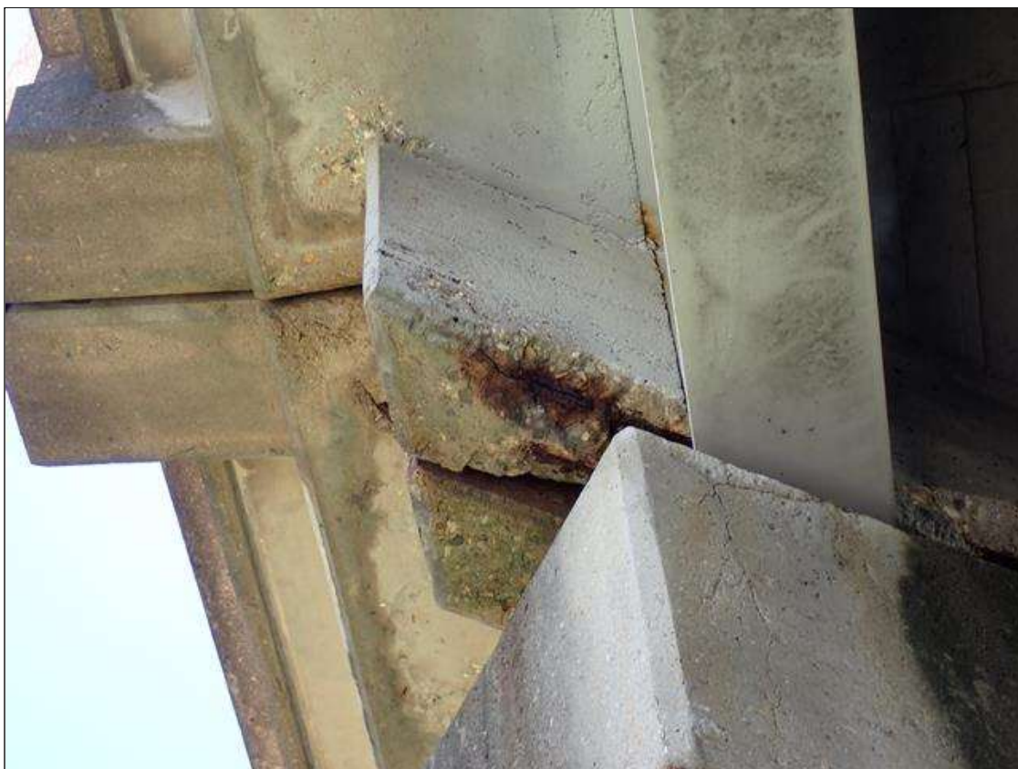
Span 3 Beam 1: (PAR) 16 INCH X 10 INCH X 6 INCH DIAPHRAGM SPALL WITH EXPOSED REINFORCING WEST OVERHANG AT BENT 3
