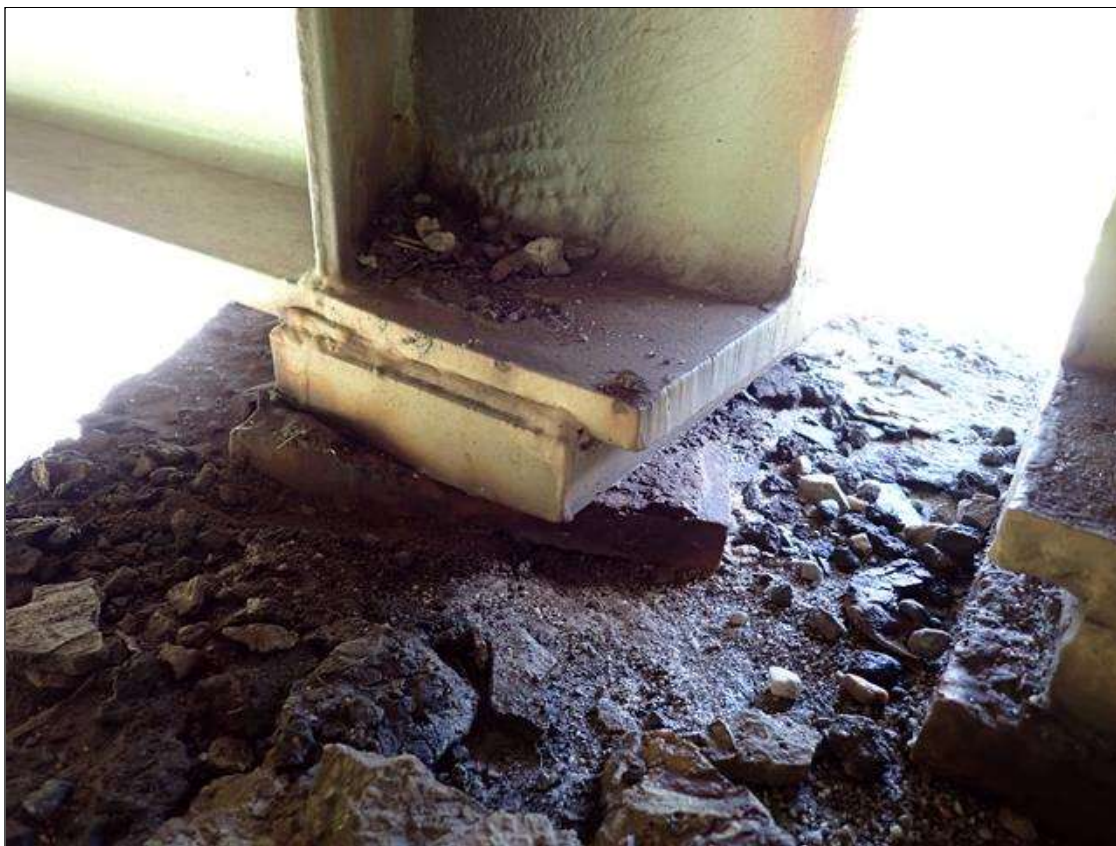
Span 3 Beam 4 - Near Bearing 4: [PAR] right and left attachment bolt sheared, masonry plate rotated
