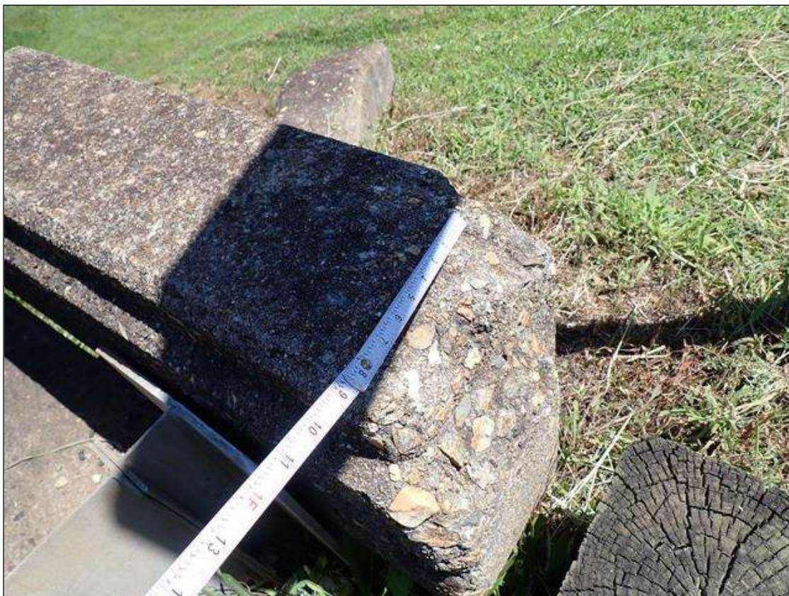
Span 1 Right Bridge Rail: at Southeast corner, spall [5 inch x full width x 1/2 inch deep]
