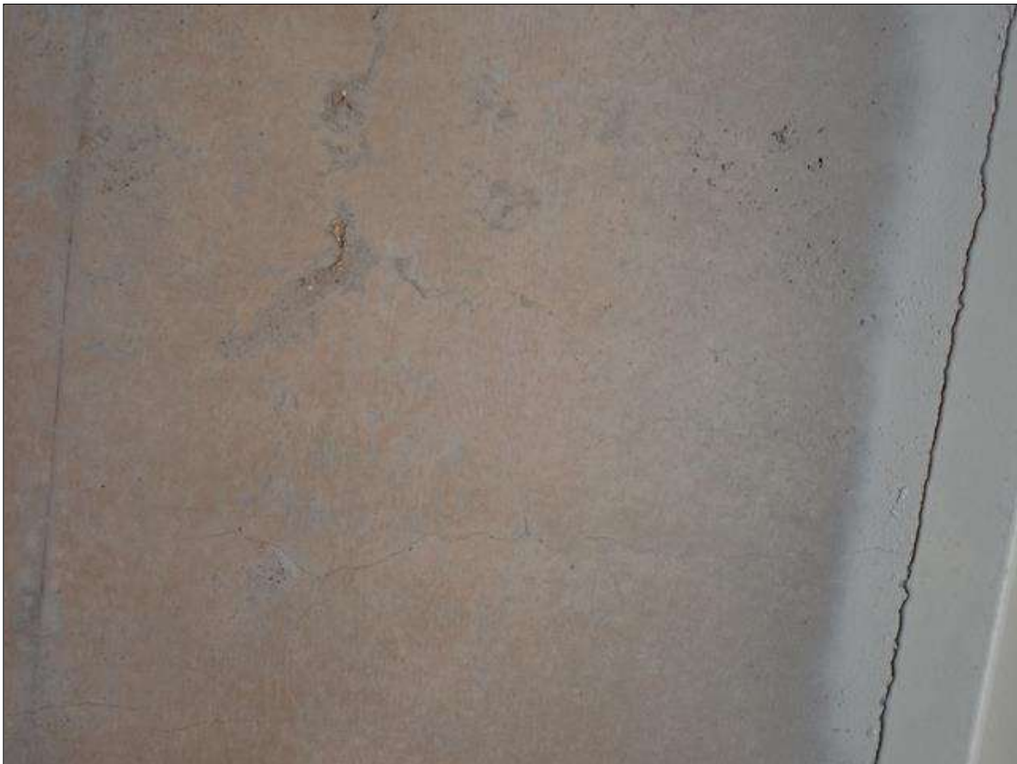
Span 3 Deck: SPAN 3 BOTTOM OF DECK HAS SCATTERED MAP CRACKS HAIRLINE AND TRANSVERSE CRACKS UP 1/32 INCH X FULL WIDTH
