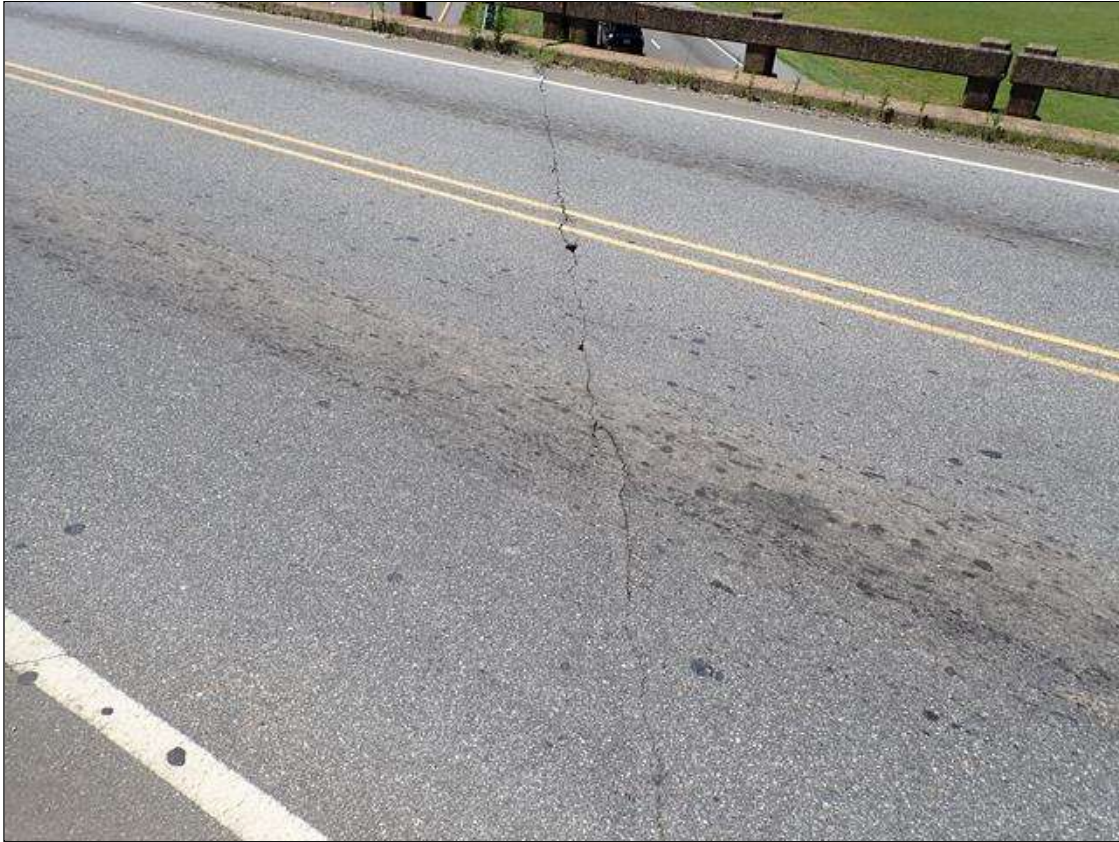
Span 2 Wearing Surface: 32 FOOT X UP TO 1/4 INCH TRANSVERSE CRACKS OVER BENT 2 WITH MULTIPLE AREAS OF BROKEN ASPHALT
