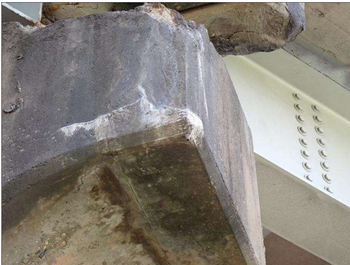
Bent 2 Cap 1: (PAR) CRACKED PATCHED AREA SOUTHEAST BOTTOM CORNER WITH EFFLORESCENCE BUILD-UP
