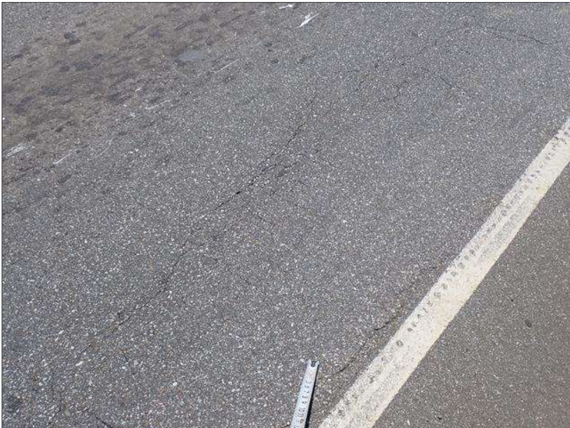
Span 1 Wearing Surface: scattered throughout, multiple transverse and longitudinal cracks [up to 6 foot x up to 1/32 inch]
