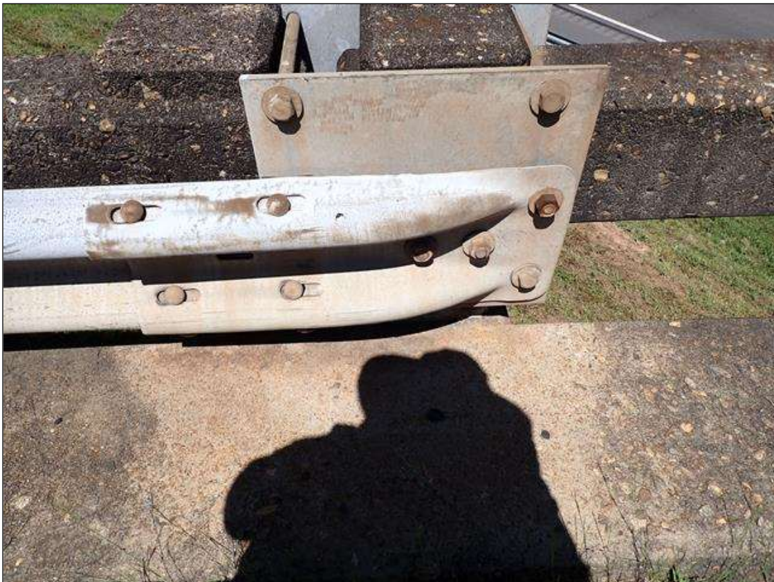
southwest guardrail attachment
