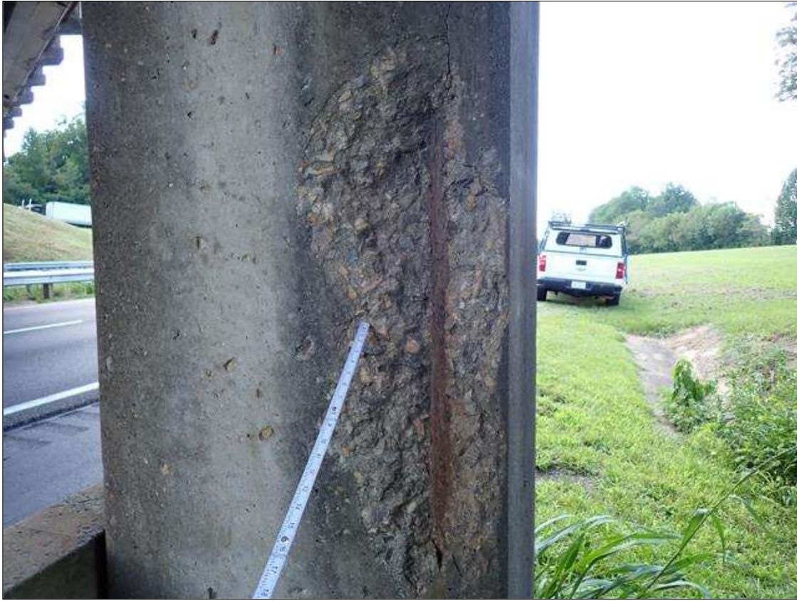
Bent 3 Pile 1: (PAR) 34 INCH X UP TO 13 INCH X 1.5 INCH DEEP SPALL WITH EXPOSED REINFORCING APPROXIMATELY 25 PERCENT LOSS, 8 FOOT FROM BOTTOM OF CAP EAST FACE
