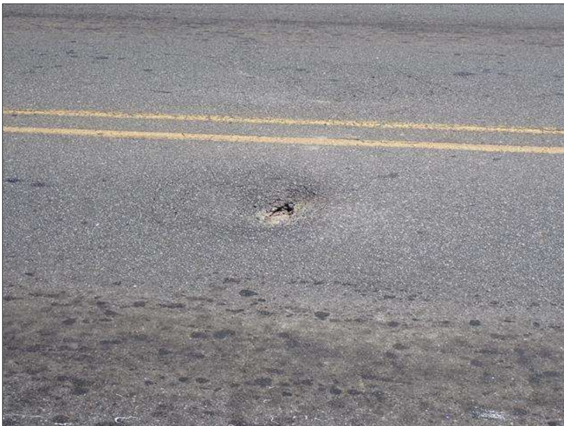
Span 1 Wearing Surface: near midspan, southbound lane, pothole/broken asphalt [5 inch x 11 inch x up to 1 inch deep]
