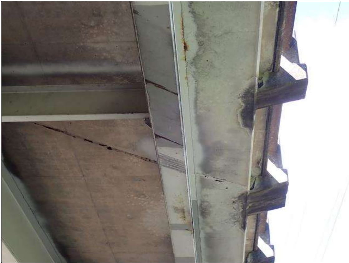
Span 2 Beam 4: underside of coverplate over right travel lane, impact scrapes with surface rust
