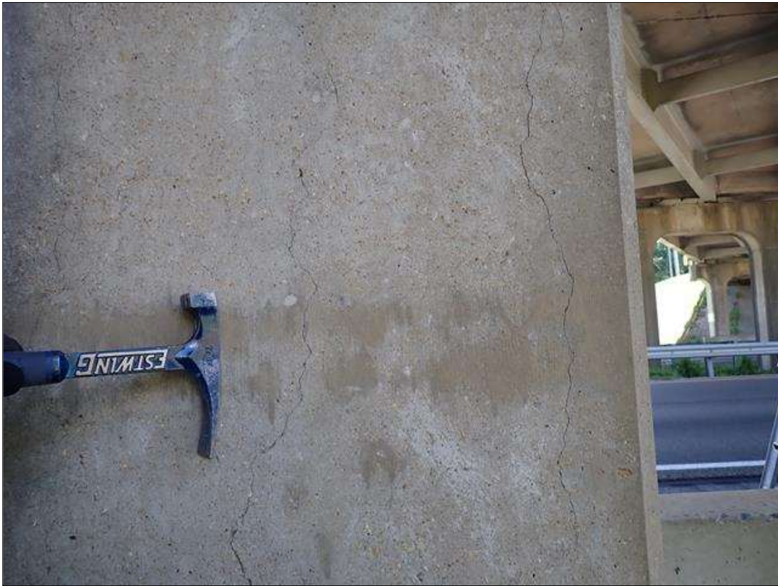
Bent 3 Pile 2: all faces, multiple vertical cracks [1/32 inch x full height]
