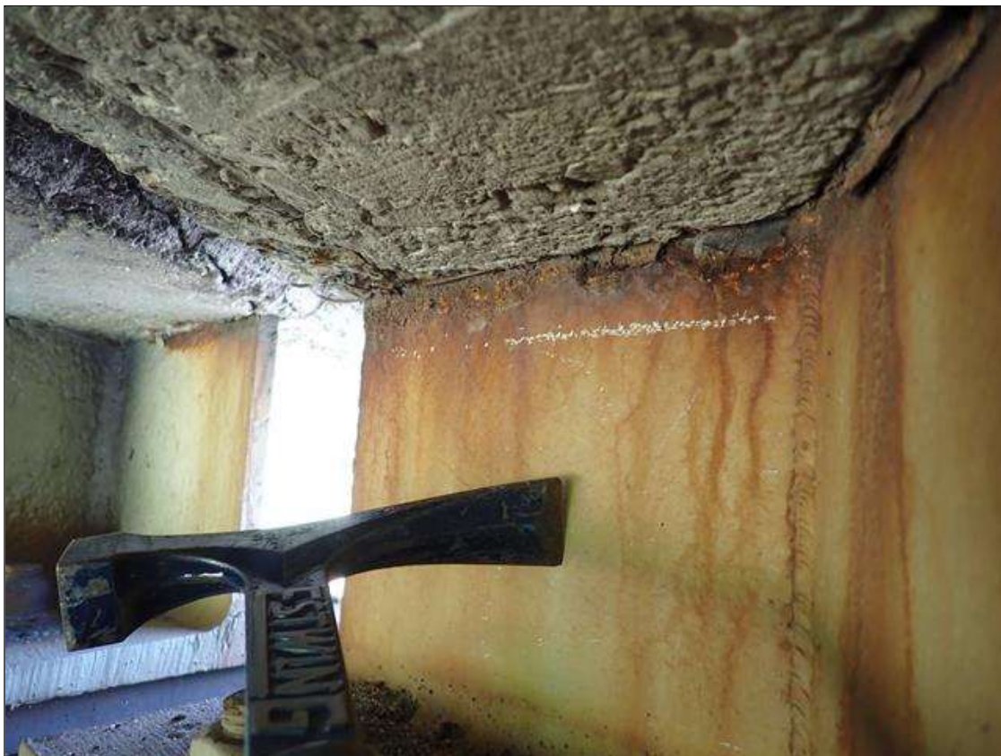
Span 3 Beam 4: at bent 3, web adjacent to diaphragm, rust scale (10 inch)
