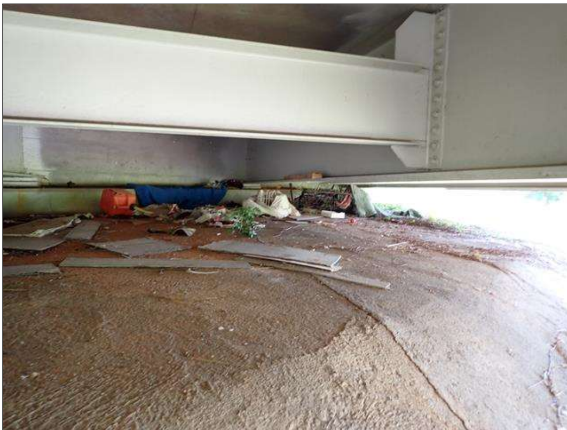
at end bent 2, slope protection, homeless debris
