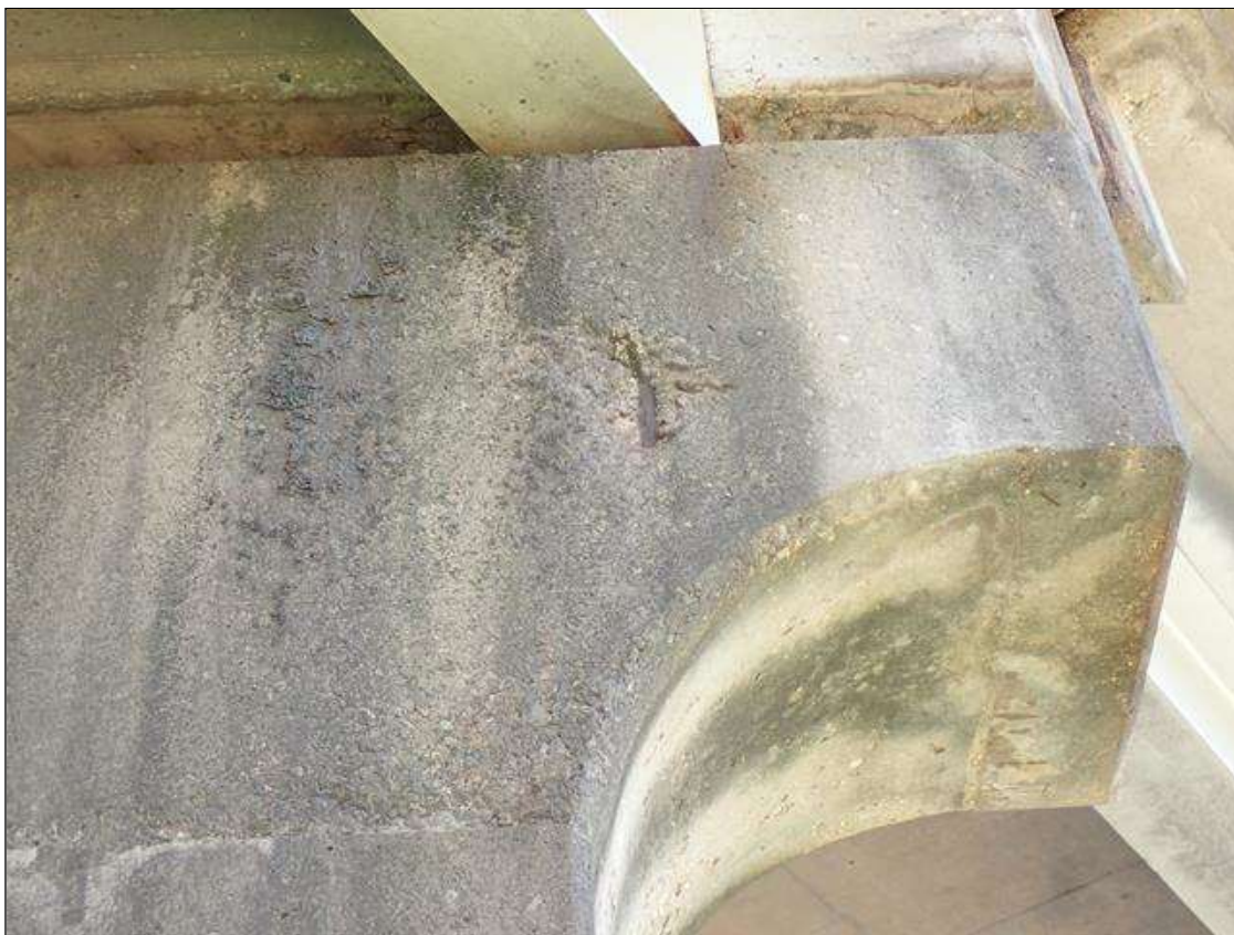
Bent 3 Cap 1: (PAR) North face below beam 1, spall [13 inch x 15 inch x 1 inch deep] with exposed rusted reinforcing [section loss up to 1/16 inch]
