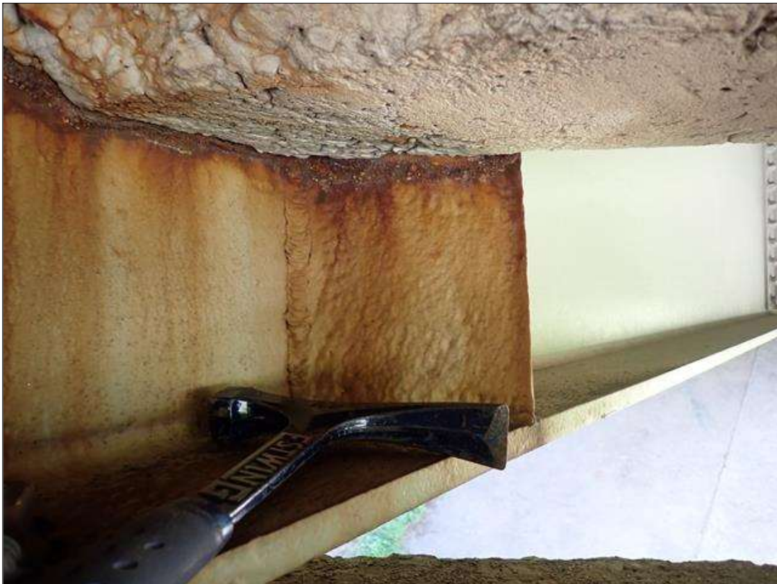
Span 1 Beam 2: at bent 1, corrosion with section loss: web adjacent to diaphragm (1/2 inch average remaining x 10 inch x 5 inch); left stiffener (0.35 inch average remaining x full width x full height)
