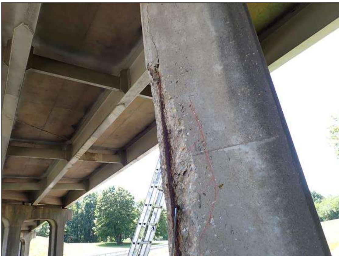
Bent 3 Pile 2: [PAR] at Southeast corner, spall [8.5 foot x 11 inch x 2.5 inch deep] with exposed rusted reinforcing [section loss up to 1/8 inch]
