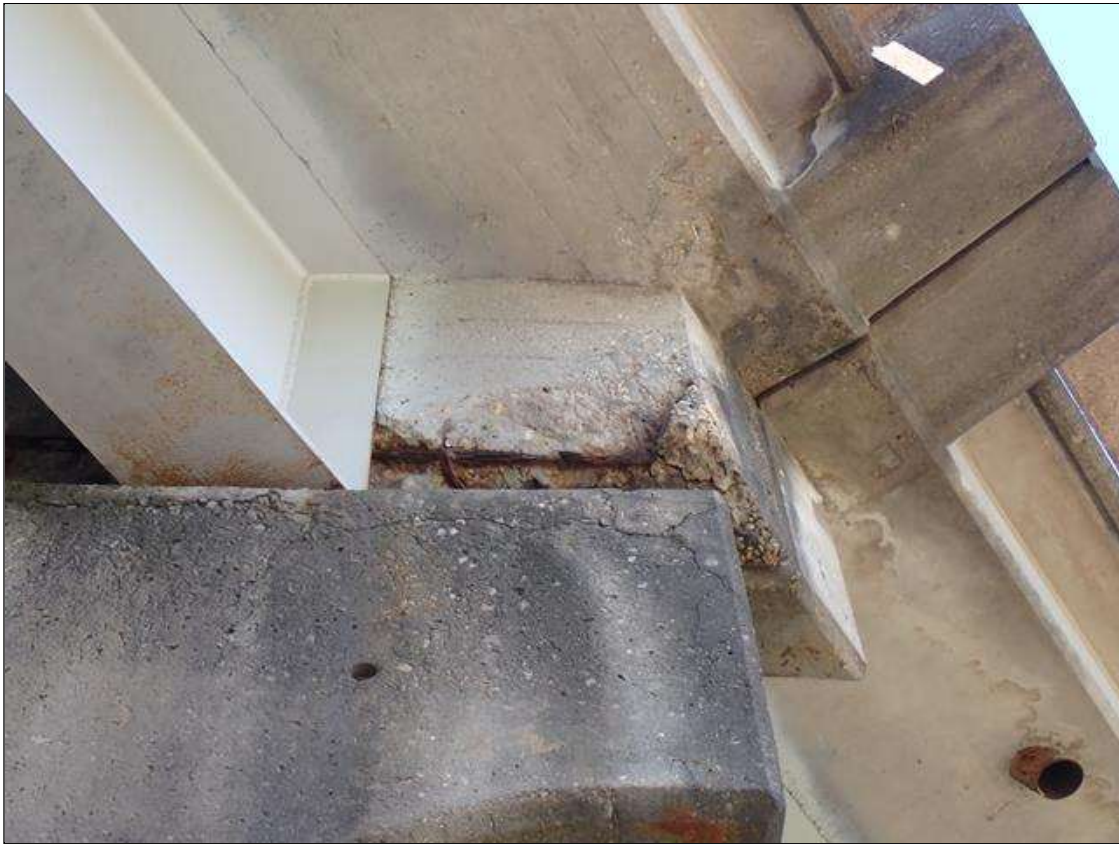
Span 3 Beam 4: (PAR) 2 FOOT X 10 INCH X 8 INCH DIAPHRAGM SPALL WITH EXPOSED REINFORCING APPROXIMATELY 25 PERCENT LOSS, EAST OVERHANG AT BENT 3
