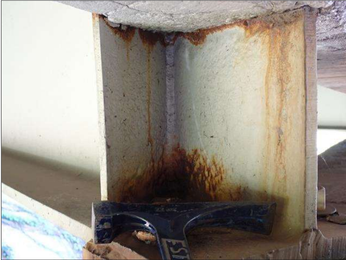
Span 4 Beam 3: at near end, arrested metal loss with corrosion reactivating, web at diaphragm [10 inch x 1 inch x 9/16 inch average remaining]; lower web, pitting [10 inch x 3 inch x up to 1/16 inch deep]; left stiffener, pitting [up to 1/8 inch deep x full width x 4 inch]
