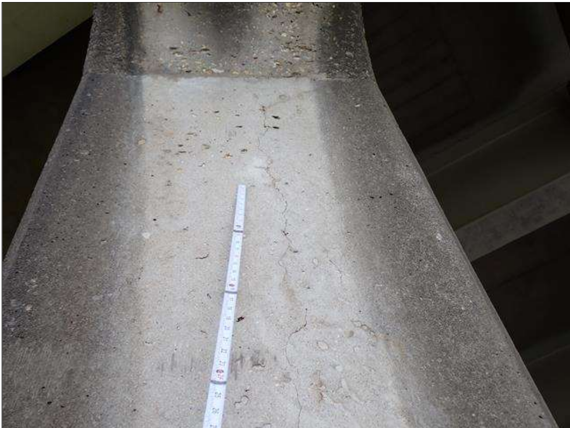
Bent 3 Pile 1: at East and West face, multiple vertical cracks [up to 8 foot x up to 1/32 inch]
