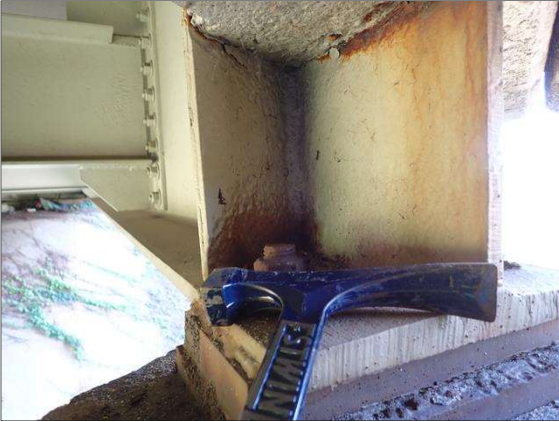
Span 4 Beam 4: at near end, arrested metal loss with corrosion reactivating: web at diaphragm [10 inch x 1/2 inch x 9/16 inch average remaining]; left stiffener [0.30 inch average remaining x full width x full height]; lower web, pitting [up to 1/16 inch deep x 10 inch x 3 inch]
