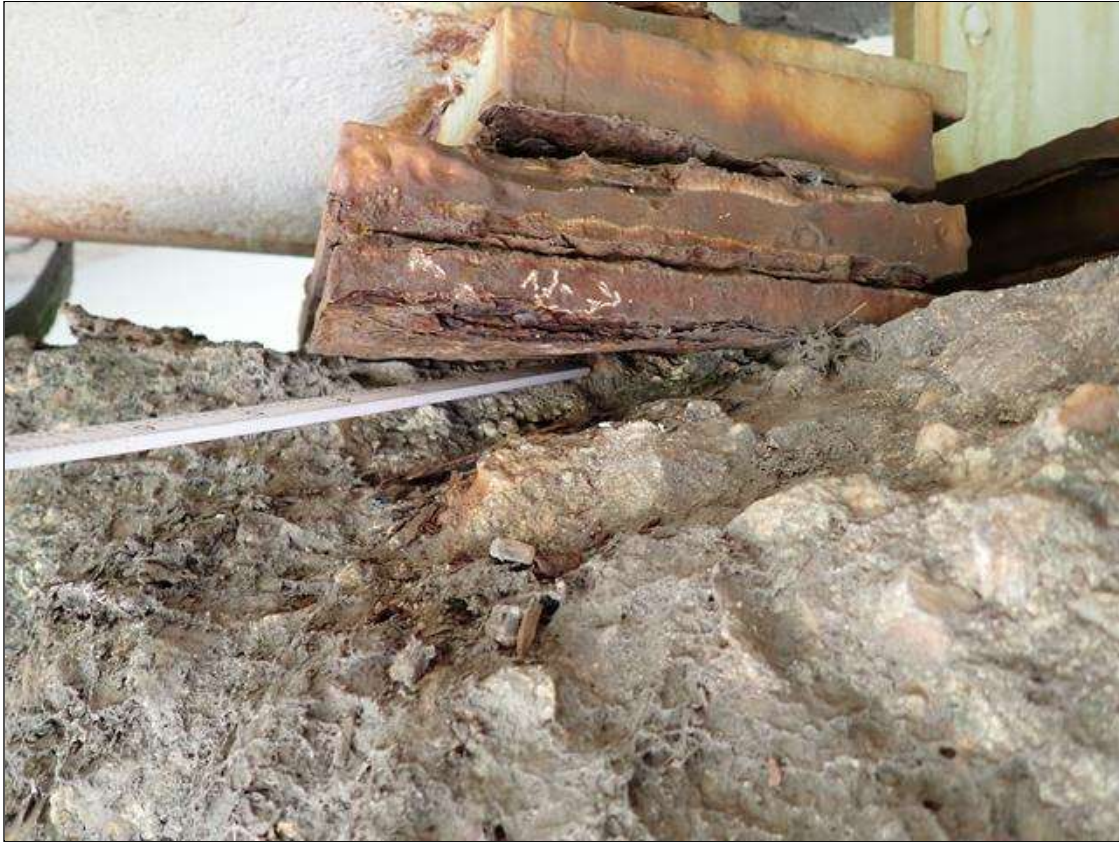
Span 3 Beam 2 - Near Bearing 2: [PAR] SPAN 3 BEAM 2 NEAR BEARING NORTHWEST CORNER HAS 5 INCH X 3 INCH X 4 INCH DEEP AREA OF BEARING LOSS. DUE TO BENT 2 CAP SPALLED AREA.
