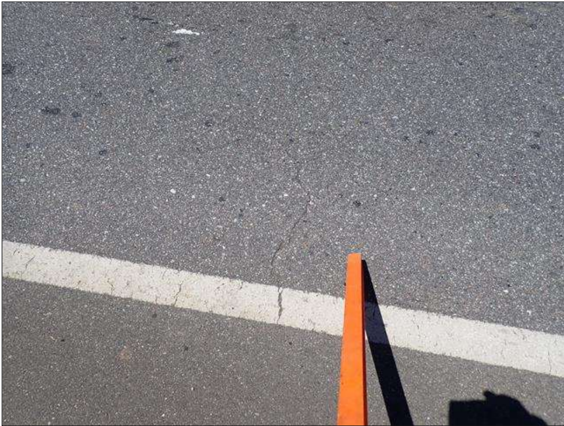
Span 2 Wearing Surface: scattered throughout, multiple transverse and longitudinal cracks [up to 4 foot x up to 1/32 inch]
