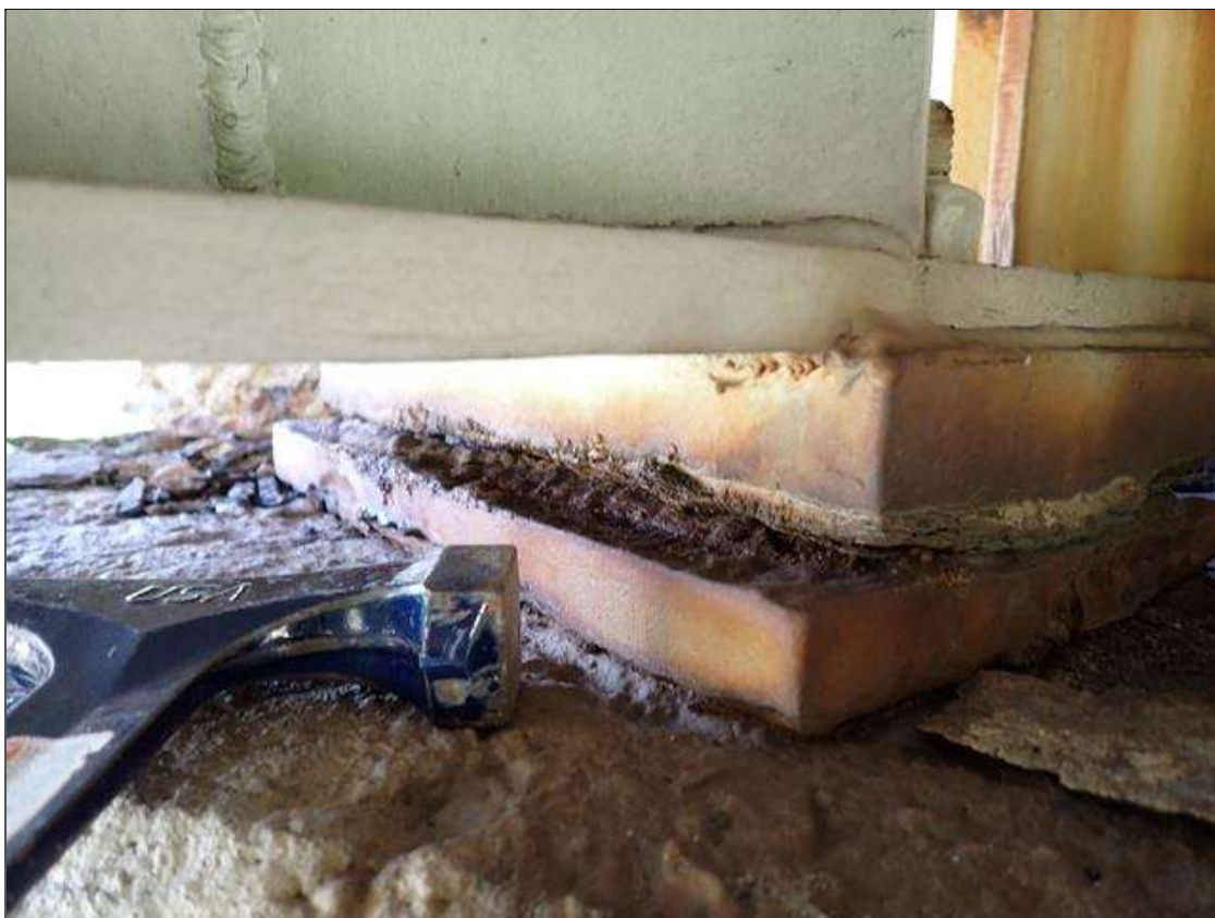
Span 3 Beam 1 - Far Bearing 1: corrosion with section loss (up to 1/8 inch loss) with pack rust (up to 3/8 inch)
