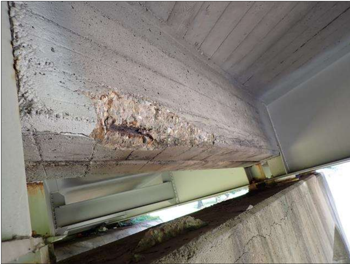
Span 3 Beam 2: (PAR) 4 FOOT X 10 INCH X 6 INCH X 2.5 INCH DEEP DIAPHRAGM SPALL/DELAMINATION WITH EXPOSED REINFORCING APPROXIMATELY 25 PERCENT LOSS, BAY 2 OVER BENT 3
