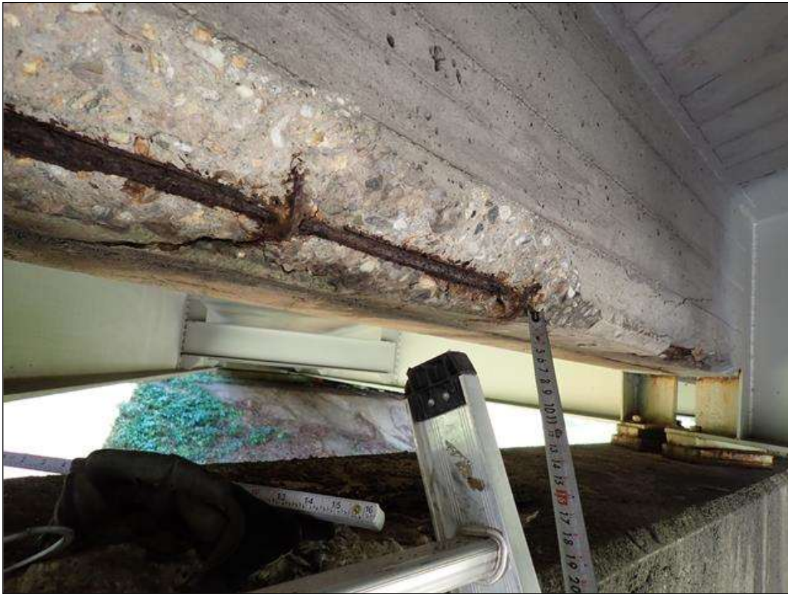
Span 3 Beam 1: (PAR) UP TO 8 FOOT X 10 INCH X 2 INCH DIAPHRAGM SPALL/DELAMINATION WITH EXPOSED REINFORCING APPROXIMATELY 25 PERCENT LOSS, BAY 1 OVER BENT 3
