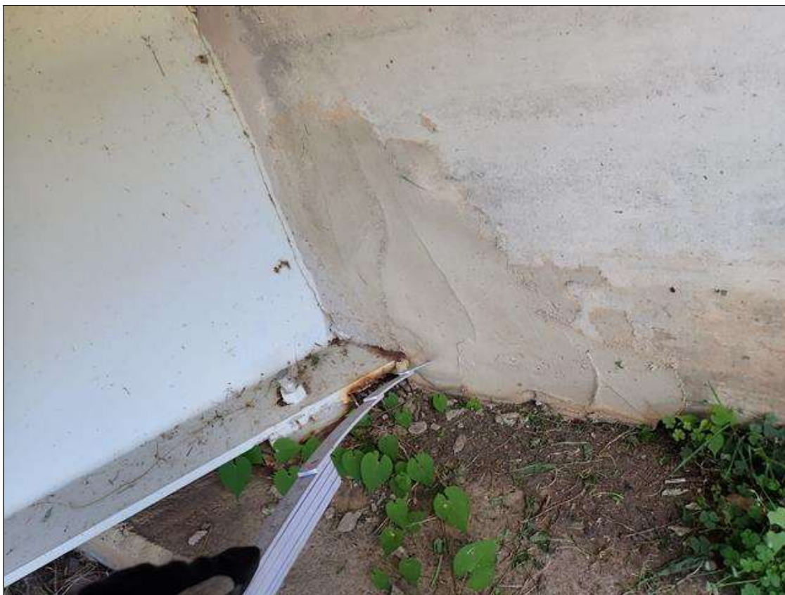
End Bent 1 Abutment: 16 INCH X UP TO 20 INCH PATCH WEST OVERHANG OF ABUTMENT
