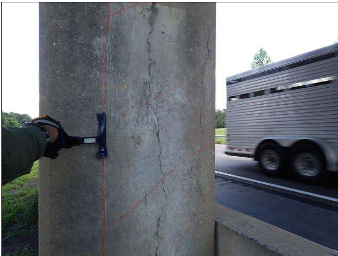
Bent 3 Pile 2: 2 - VERTICAL CRACKS UP TO 9 FOOT X 1/16 INCH WITH ADJACENT DELAMINATION 9 FOOT X 2 FOOT ON WEST FACE
