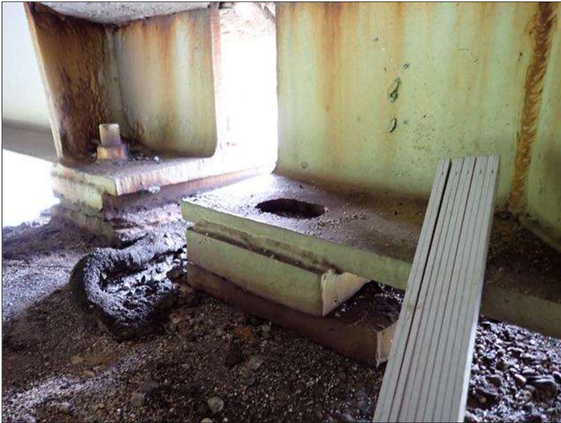
Span 3 Near Bearing 1: [PAR] right and left attachment bolt sheared
