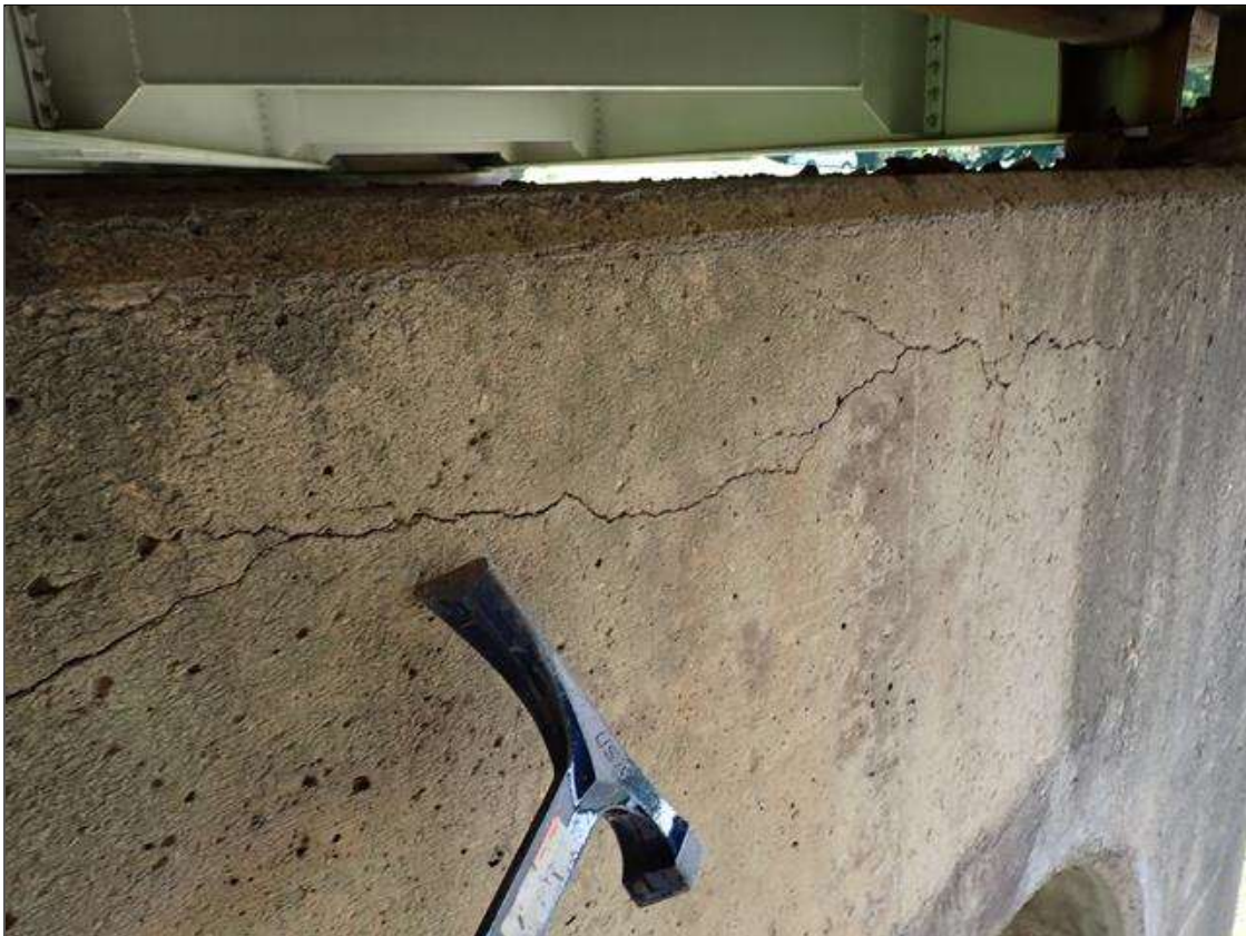
Bent 1 Cap 1: MAP CRACKING AND HORIZONTAL CRACKS UP TO 1/16 INCH AT RANDOM THROUGHOUT NORTH AND SOUTH FACES
