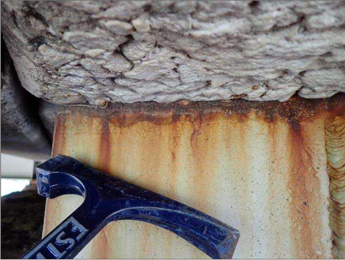
Span 2 Beam 1: at bent 2, corrosion with section loss: web adjacent to diaphragm (1/2 inch average remaining x 10 inch x 1 inch); right stiffener (0.30 average remaining x full width x full height)
