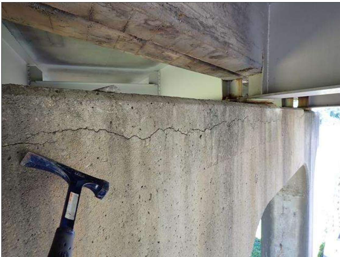
Bent 3 Cap 1: along the length of the cap, near top and bottom corners, horizontal cracks (up to 1/8 inch x 9 foot)
