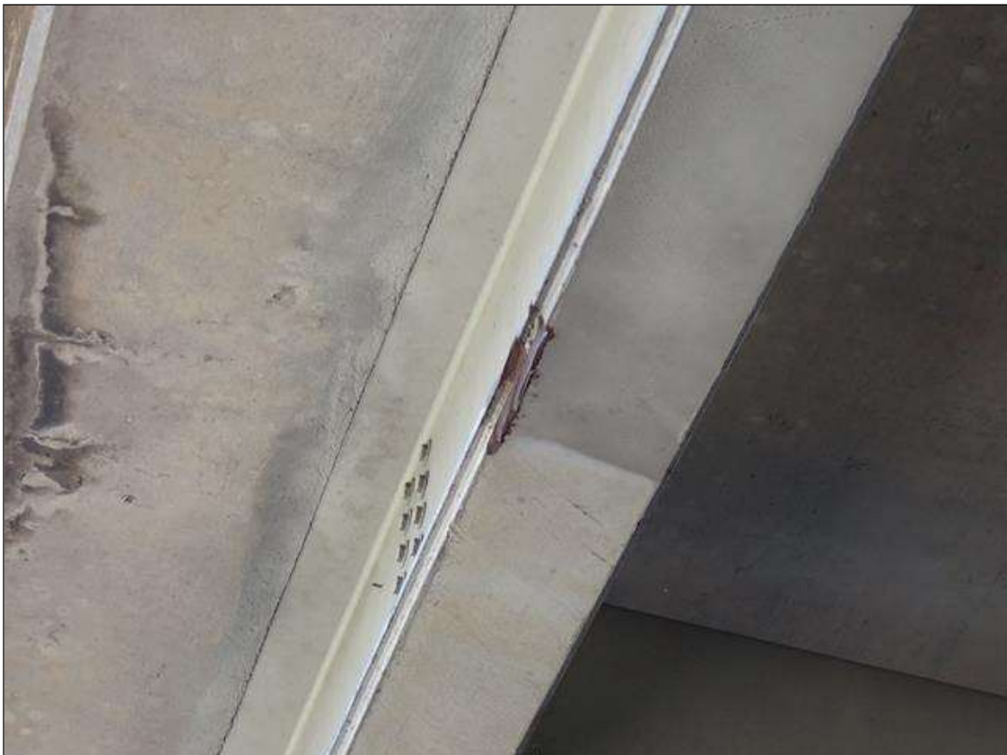
Span 3 Beam 4: (PAR) over right travel lane, impact damage with distortion (12 inch x 1 inch x 1/4 inch deep) and scrapes and surface rust
