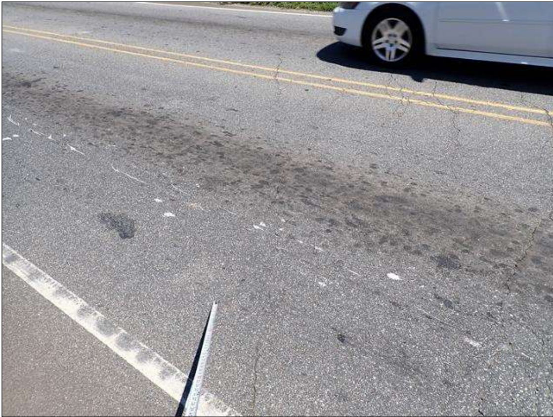
Span 1 Wearing Surface: 32 FOOT X UP TO 1/4 INCH TRANSVERSE CRACKS OVER END BENT 1 AND BENT 1 WITH VEGETATION GROWTH
