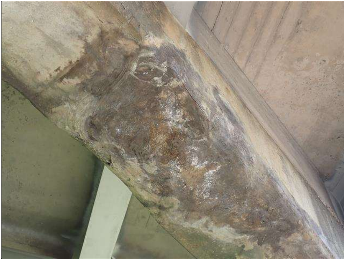
Bent 1 Cap 1: (PAR) MULTIPLE UP TO 8 FOOT X 2.5 FOOT CRACKED/FAILED PATCHED AREAS WITH EXPOSED RUSTED REBAR APPROXIMATELY 25 PERCENT LOSS, THROUGHOUT BOTTOM AND SOUTH FACE
