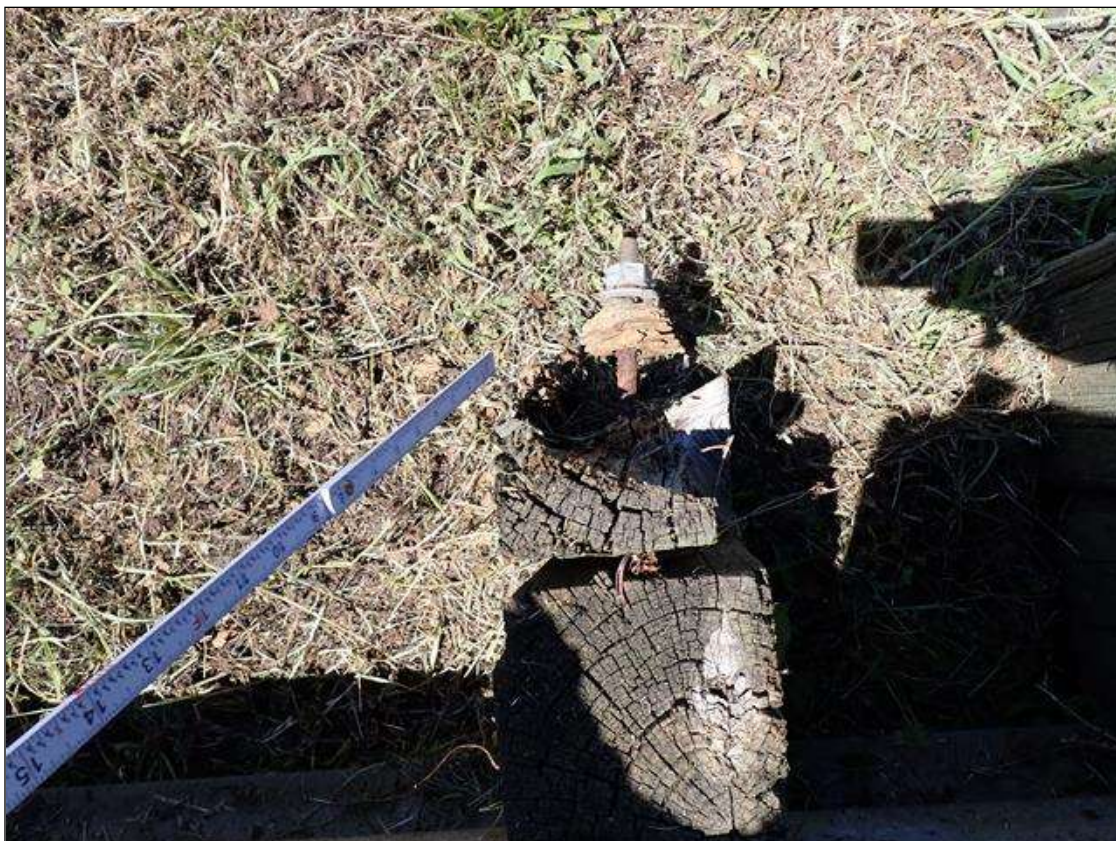
(PAR) southwest guardrail, 2nd post from end bent 1, decay (full height x full width x full depth)
