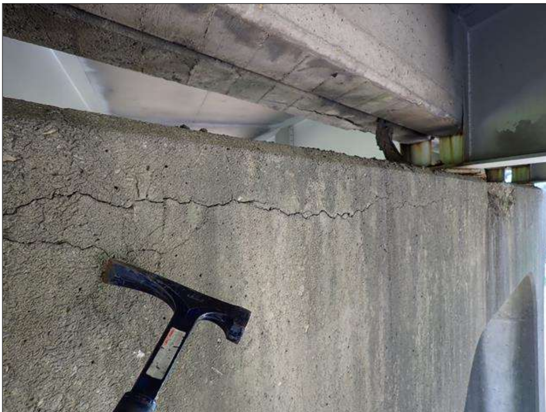
Bent 2 Cap 1: ALONG THE LENGTH OF THE CAP, SCATTERED LONGITUDINAL CRACKS UP TO 1/16 INCH
