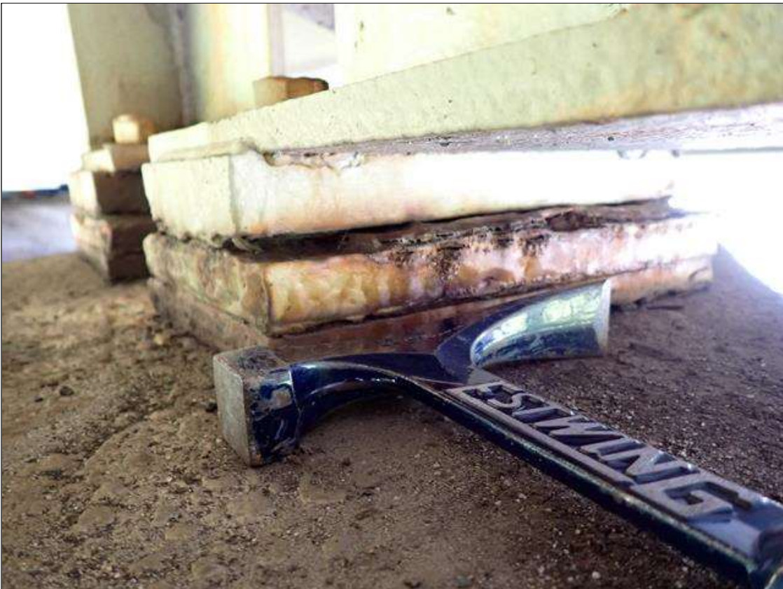
Span 3 Beam 2 - Far Bearing 2: corrosion with section loss (up to 1/16 inch deep) with pack rust (up to 3/8 inch)
