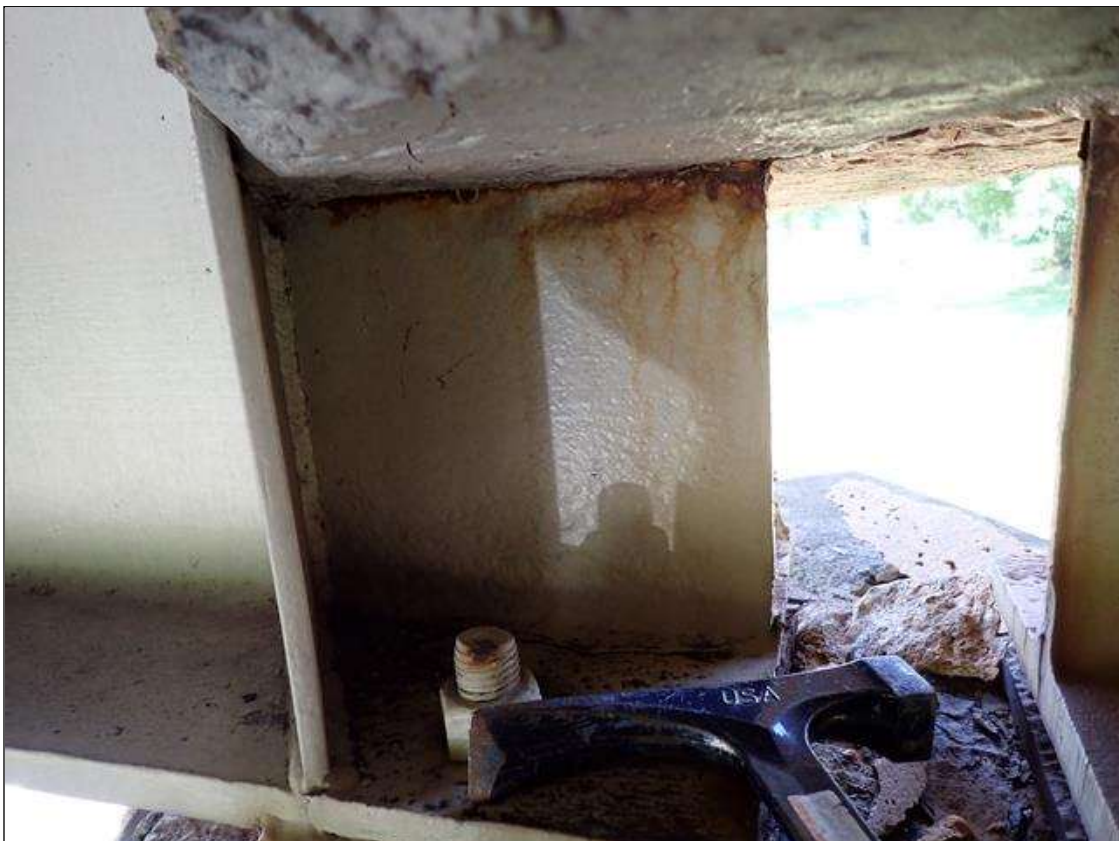
Span 3 Beam 1: at far end arrested metal loss with corrosion reactivating, web at diaphragm [10 inch x 1 inch x 1/2 inch average remaining]; arrested metal loss, lower web [8 inch x 1.5 inch x 9/16 inch average remaining]
