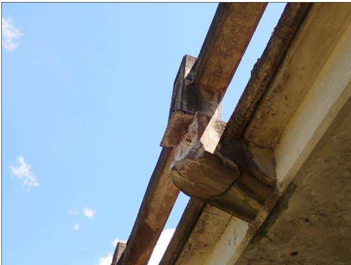
Span 1 Left Bridge Rail: [PAR] at base of rail post 8, spall [12 inch x 7 inch x up to 4 inch deep] with exposed rusted reinforcing with no loss
