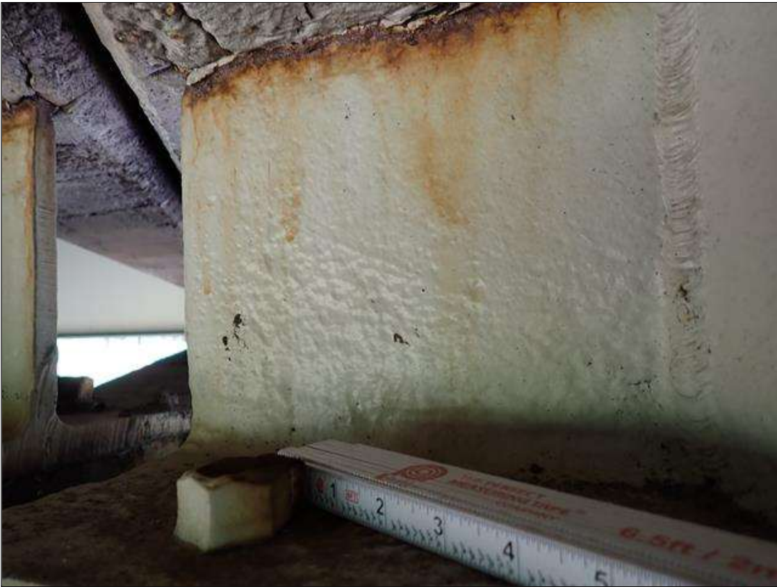
Span 3 Beam 2: at far end, arrested metal loss with corrosion reactivating, web at diaphragm [10 inch x 1 inch x 9/16 inch average remaining]; pitting [up to 1/8 inch deep]
