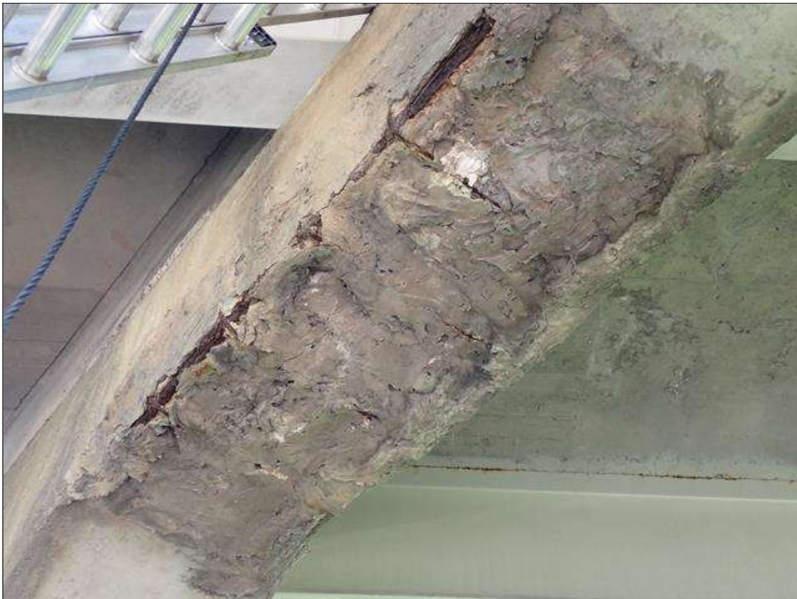
Bent 1 Cap 1: (PAR) MULTIPLE UP TO 8 FOOT X 2.5 FOOT CRACKED/FAILED PATCHED AREAS WITH EXPOSED RUSTED REBAR APPROXIMATELY 25 PERCENT LOSS, THROUGHOUT BOTTOM AND SOUTH FACE
