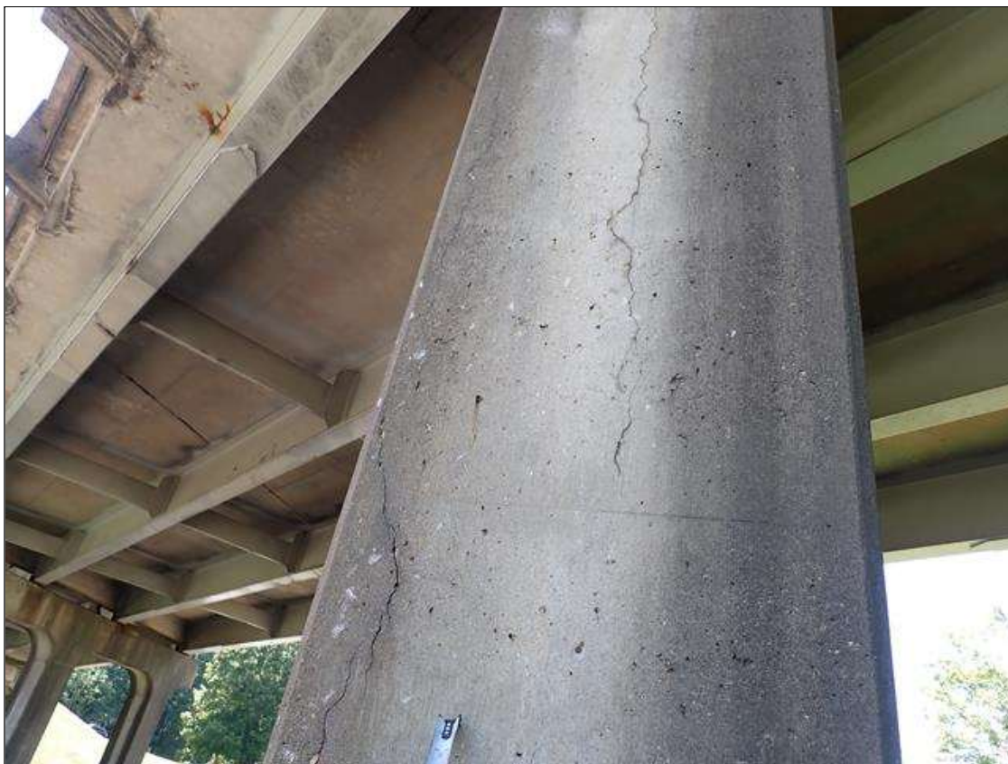
Bent 3 Pile 3: East face, multiple vertical cracks (up to full height x 1/8 inch wide) with adjacent delamination (up to full height x 1.5 foot)
