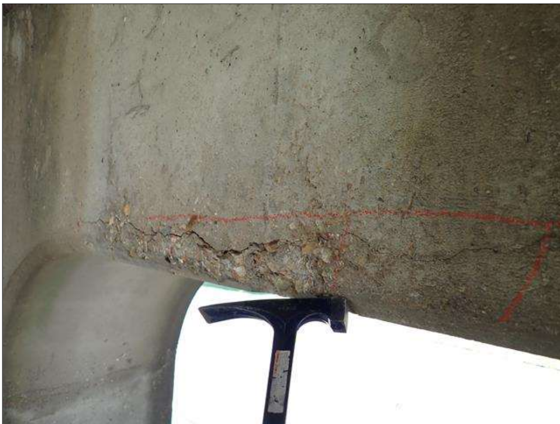
Bent 2 Cap 1: North face below beam 3, delamination [29 inch x 3 inch] with cracks [up to 1/16 inch]
