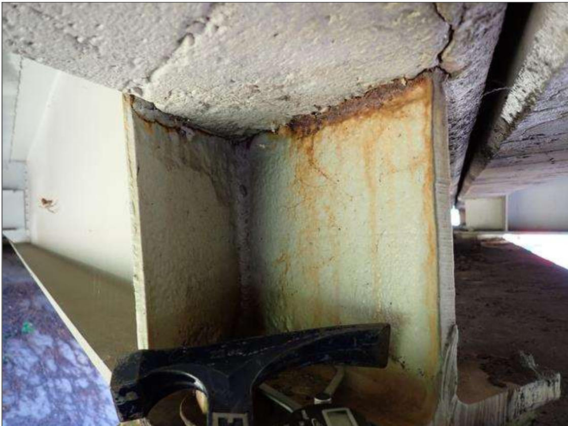
Span 4 Beam 2: at near end, arrested metal loss with corrosion reactivating, web at diaphragm [10 inch x 1/2 inch x 1/2 inch average remaining]; left stiffener [0.35 average remaining x full width x full height]
