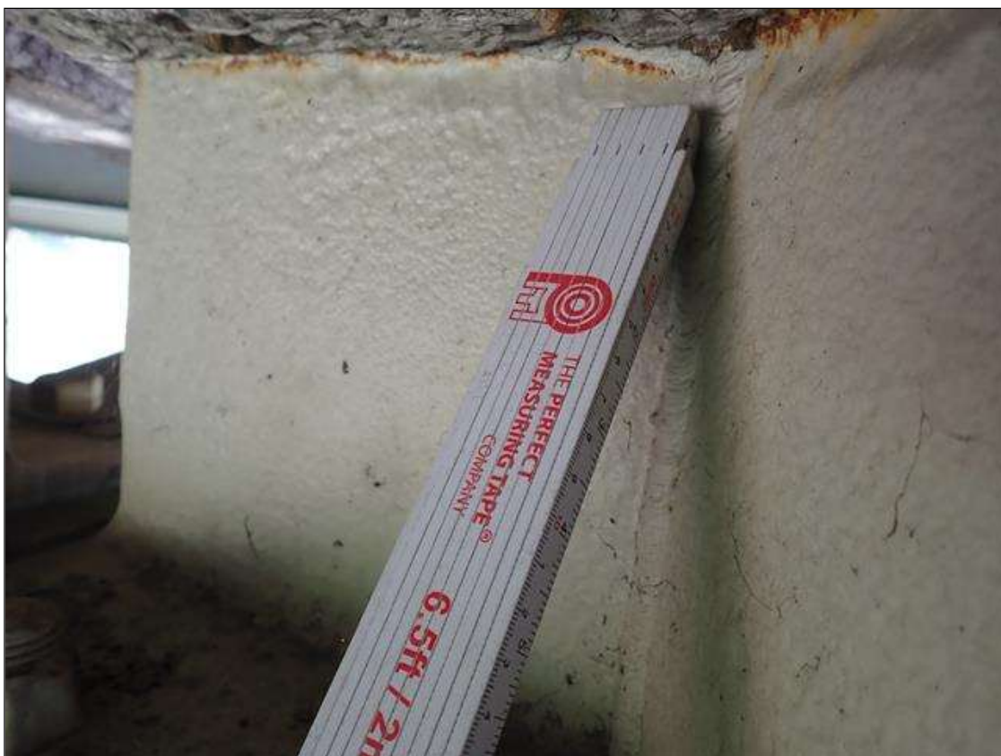
Span 3 Beam 3: at far end arrested metal loss/pitting with corrosion reactivating, web at diaphragm [10 inch x 3 inch x 1/16 inch deep]
