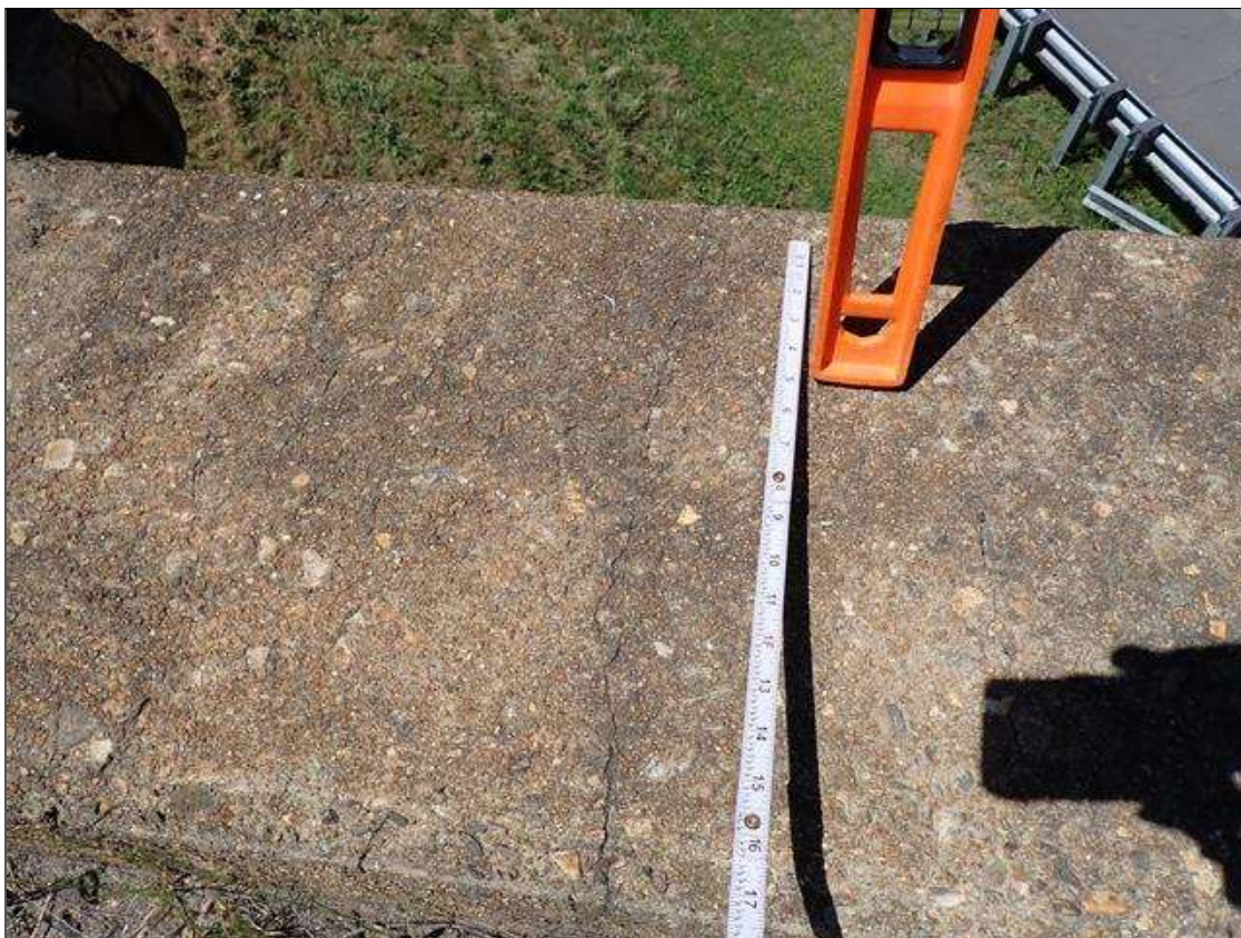
Span 1 Left Bridge Rail: along sidewalk multiple transverse cracks [up to 1/32 inch x full width]
