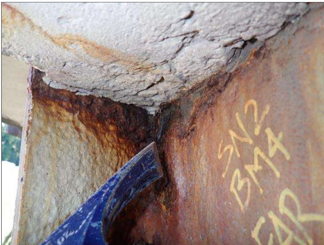
Span 2 Beam 4: [PAR] at far end, corrosion with section loss: web below diaphragm [11 inch x 2 inch x 7/16 inch average remaining]; right stiffener [0.30 inch average remaining x full width x full height]
