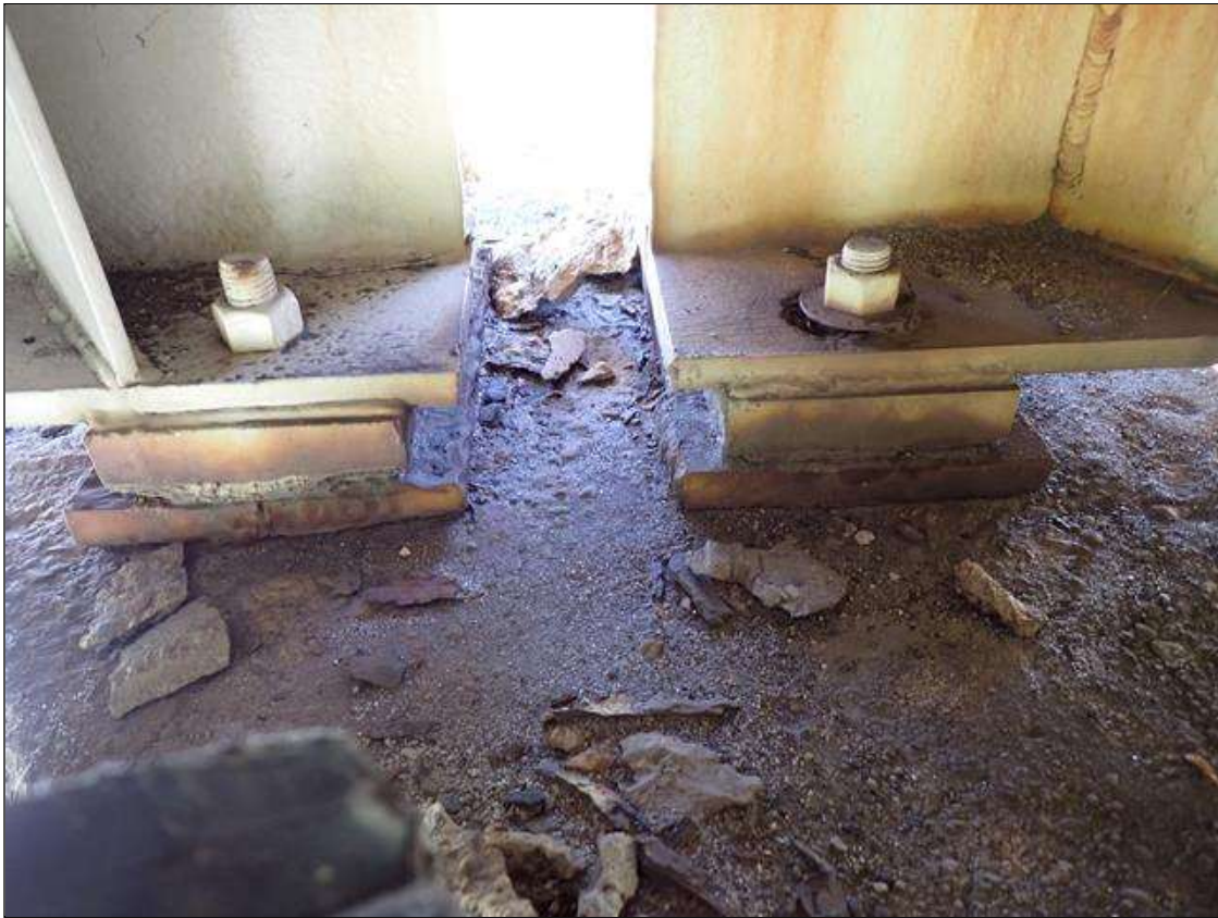
interior bearing assembly
