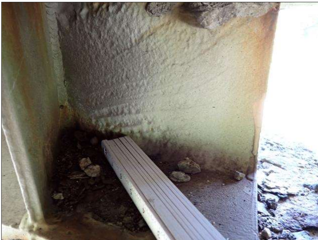
Span 3 Beam 4: at bent 2, painted over pitting: web (up to 1/8 inch deep x 10 inch x full height)
