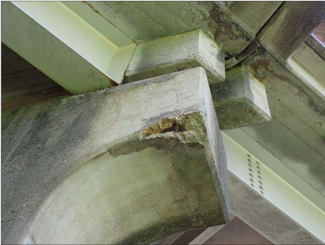
Bent 1 Cap 1: (PAR) MULTIPLE UP TO 8 FOOT X 2.5 FOOT CRACKED/FAILED PATCHED AREAS WITH EXPOSED RUSTED REBAR APPROXIMATELY 25 PERCENT LOSS, THROUGHOUT BOTTOM AND SOUTH FACE
