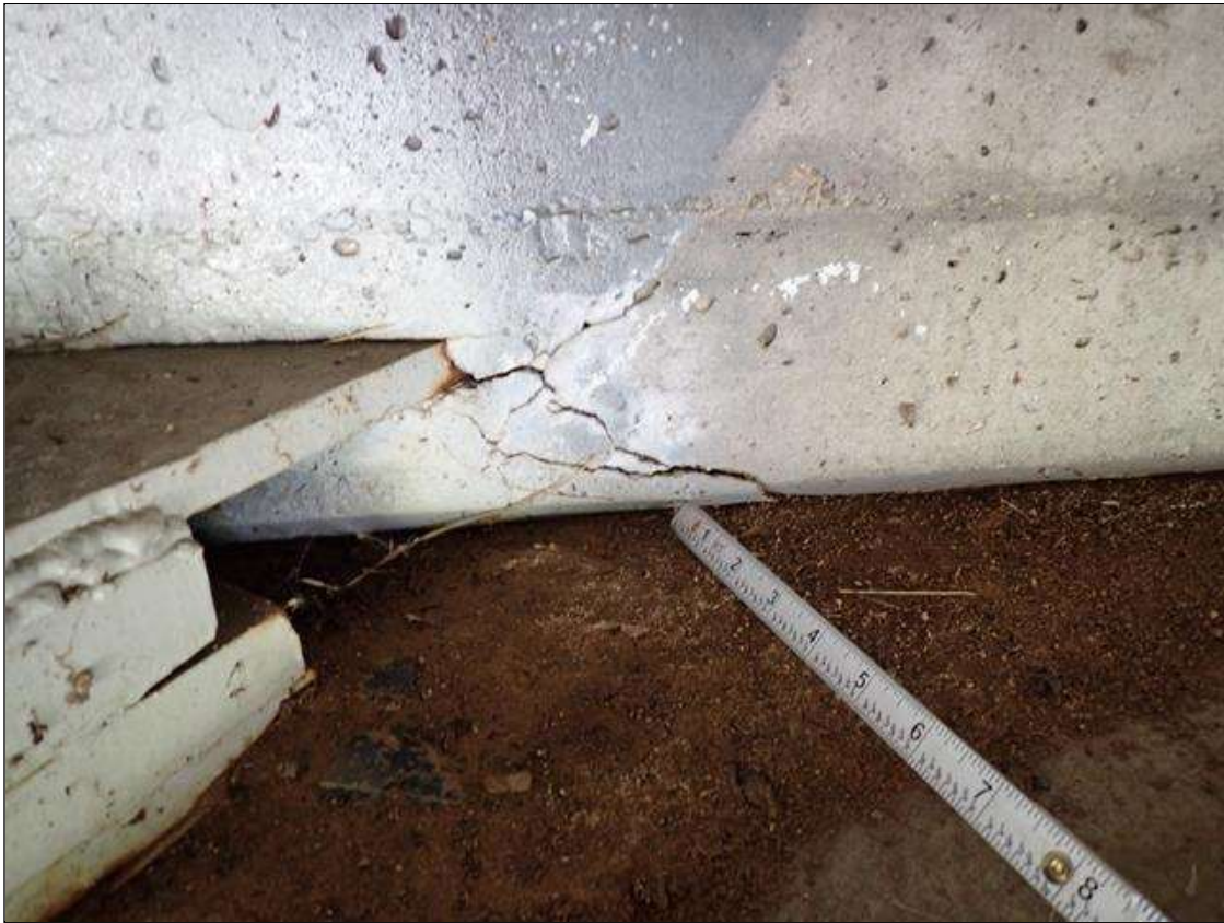
End Bent 1 Abutment: along the length of the abutment, at bottom flange penetrations, delaminations (up to 7 inch x 3 inch) with cracks (up to 1/16 inch)
