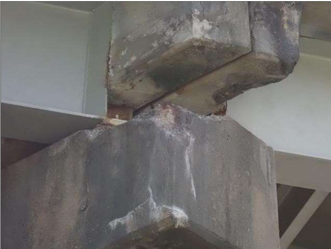
Bent 2 Cap 1: [PAR] South face at East end, corner spall [27 inch x 14 inch x 12 inch x 3 inch deep] with exposed rusted reinforcing [section loss up to 1/8 inch]
