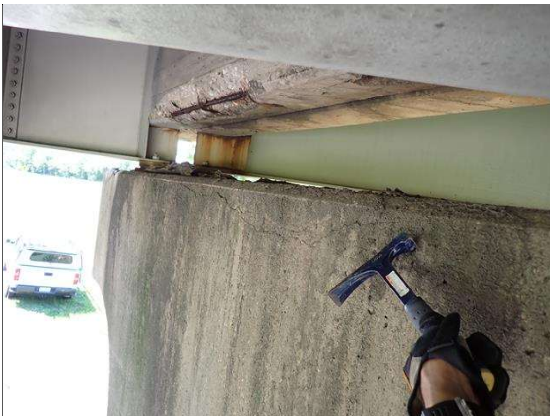
Bent 3 Cap 1: along the length of the cap, near top and bottom corners, horizontal cracks (up to 1/8 inch x 9 foot)
