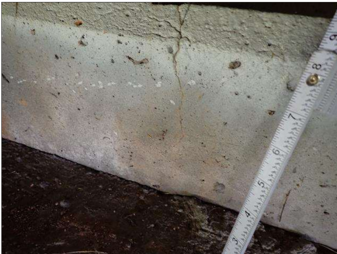
End Bent 1 Cap 1: at multiple locations throughout in all bays, wraparound vertical cracks [up to full height x 1/32 inch]
