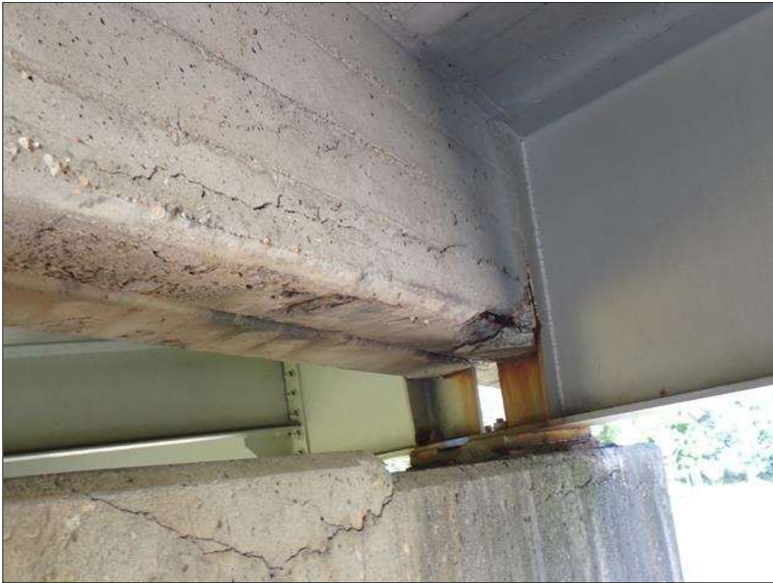
Span 3 Beam 3: (PAR) 5 FOOT X UP TO 12 INCH X 2.5 INCH DIAPHRAGM SPALL/DELAMINATION WITH EXPOSED RUSTED REBAR APPROXIMATELY 25 PERCENT LOSS, BAY 3 OVER BENT 3
