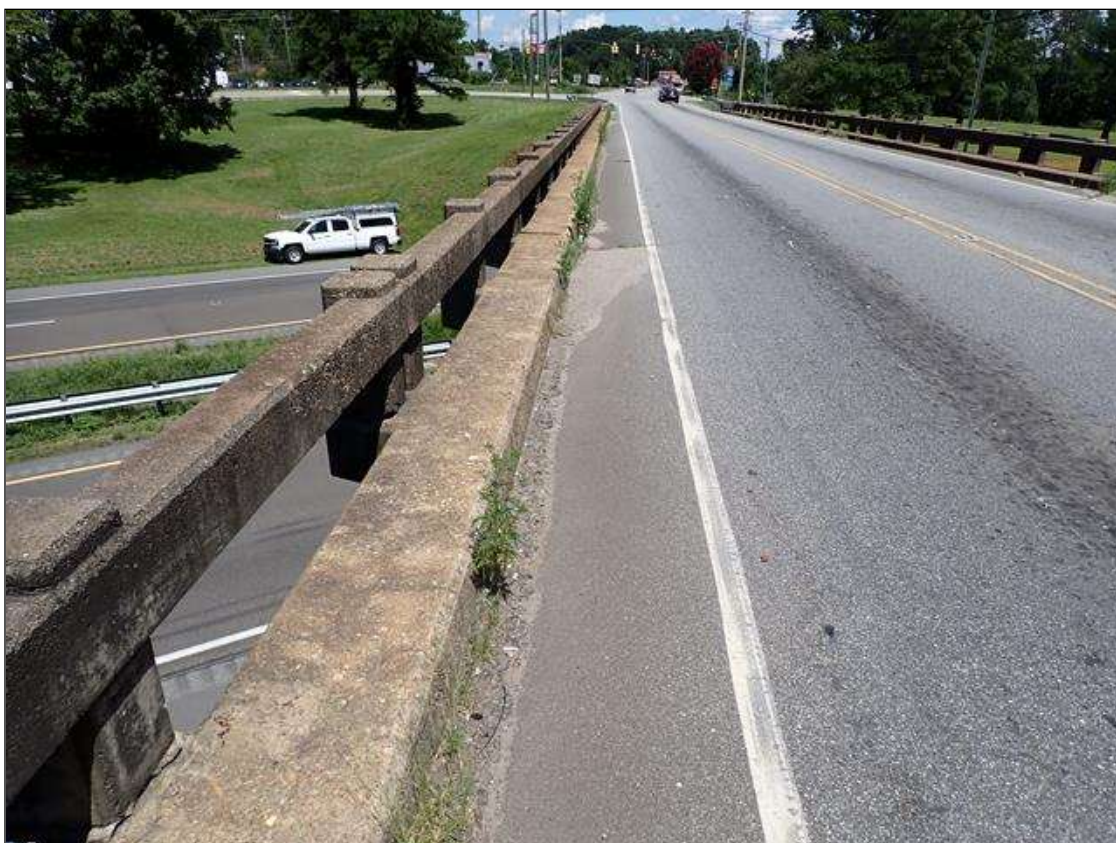
along both curblines, debris accumulation (up to 33 inch x full length) with vegetation growth; partially obstructing drainage
