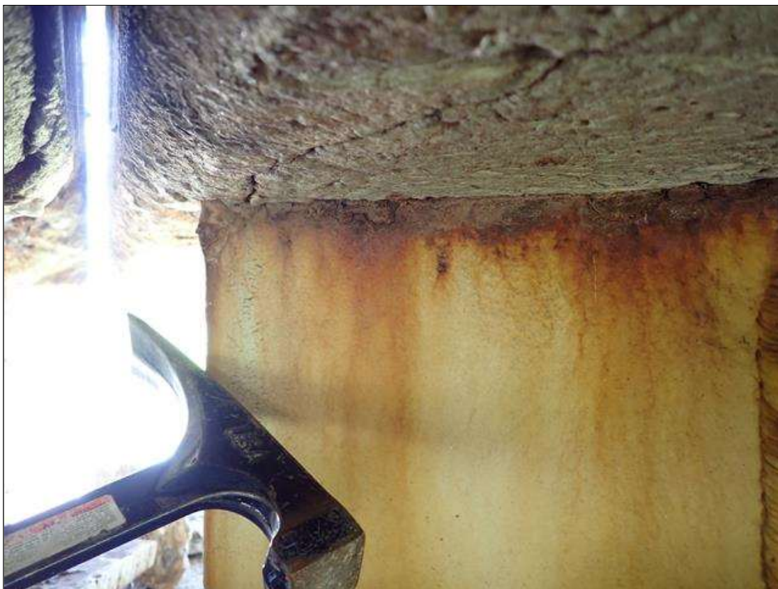
Span 4 Beam 1: at near end, arrested metal loss with corrosion reactivating, web at diaphragm [10 inch x 1/2 inch x 9/16 inch average remaining]
