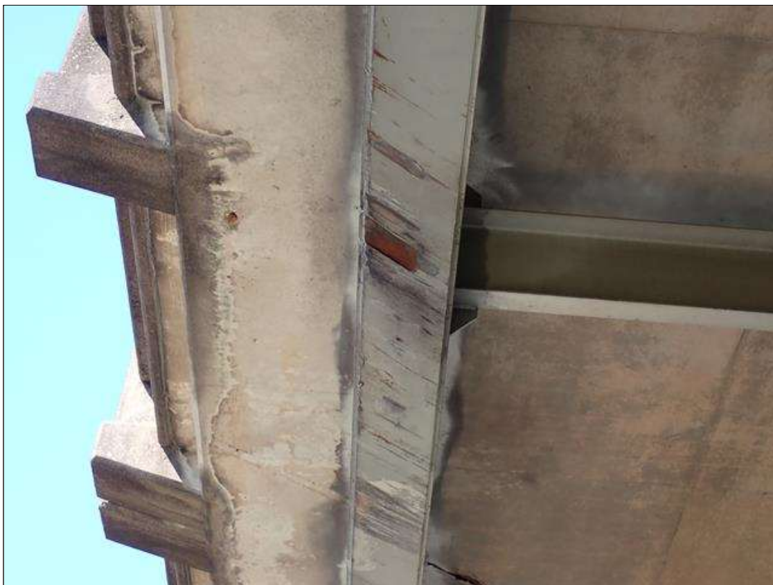
Span 2 Beam 1: (PAR) over both travel lanes, multiple vehicle impact with gouges [up to 3 inch x 1 inch x 1/2 inch deep] with surface rust
