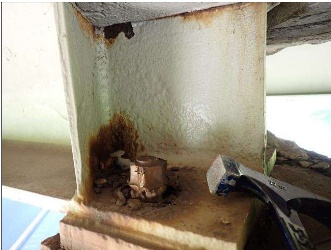
Span 3 Beam 2: at bent 2, painted over pitting with corrosion reactivating: web (up to 1/16 inch x 10 inch x full height)
