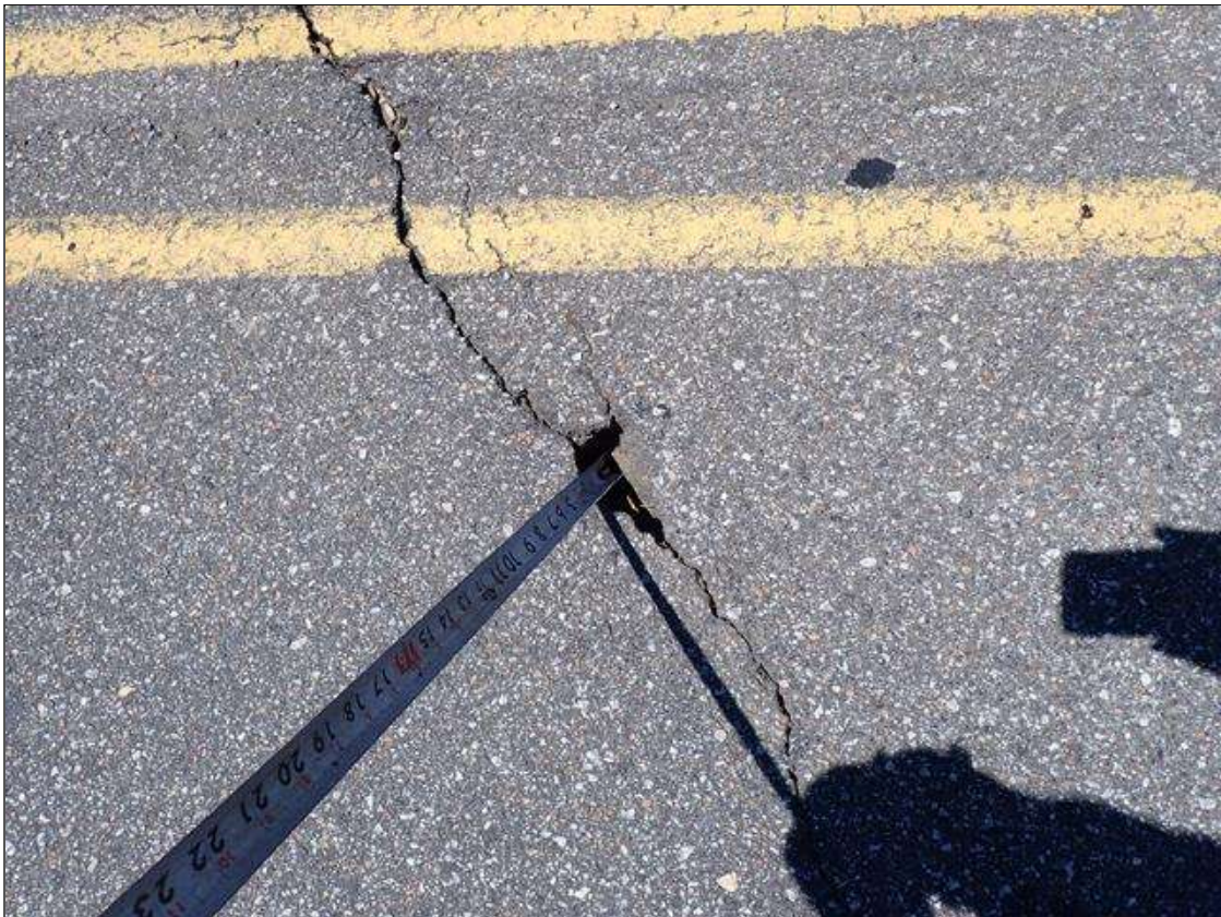
Span 2 Wearing Surface: at bent 2 beside white line in Southbound lane, pothole [9 inch x up to 3 inch x full depth] and by centerline pothole [3 inch diameter x full depth]
