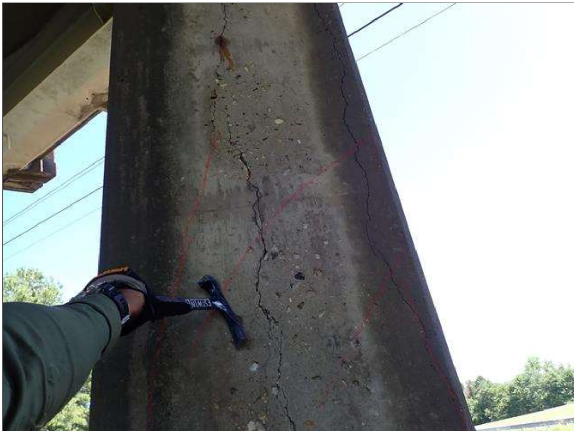
Bent 3 Pile 3: (PAR) 2 - VERTICAL CRACKS UP TO FULL HEIGHT X UP TO 1/8 INCH WITH RUST STAINS AND ADJACENT DELAMINATION FULL HEIGHT X 2 FOOT ON WEST FACE
