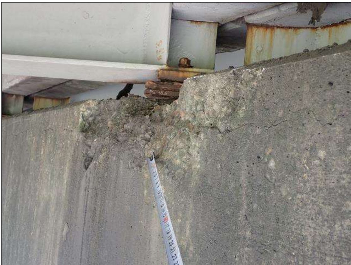
Bent 2 Cap 1: (PAR) 4 FOOT X 1 FOOT X 1 FOOT X 3 INCH DEEP CORNER SPALL WITH EXPOSED REINFORCING APPROXIMATELY 25 PERCENT LOSS, NORTH FACE UNDER BEAM 2; UNDERMINING BEARING
