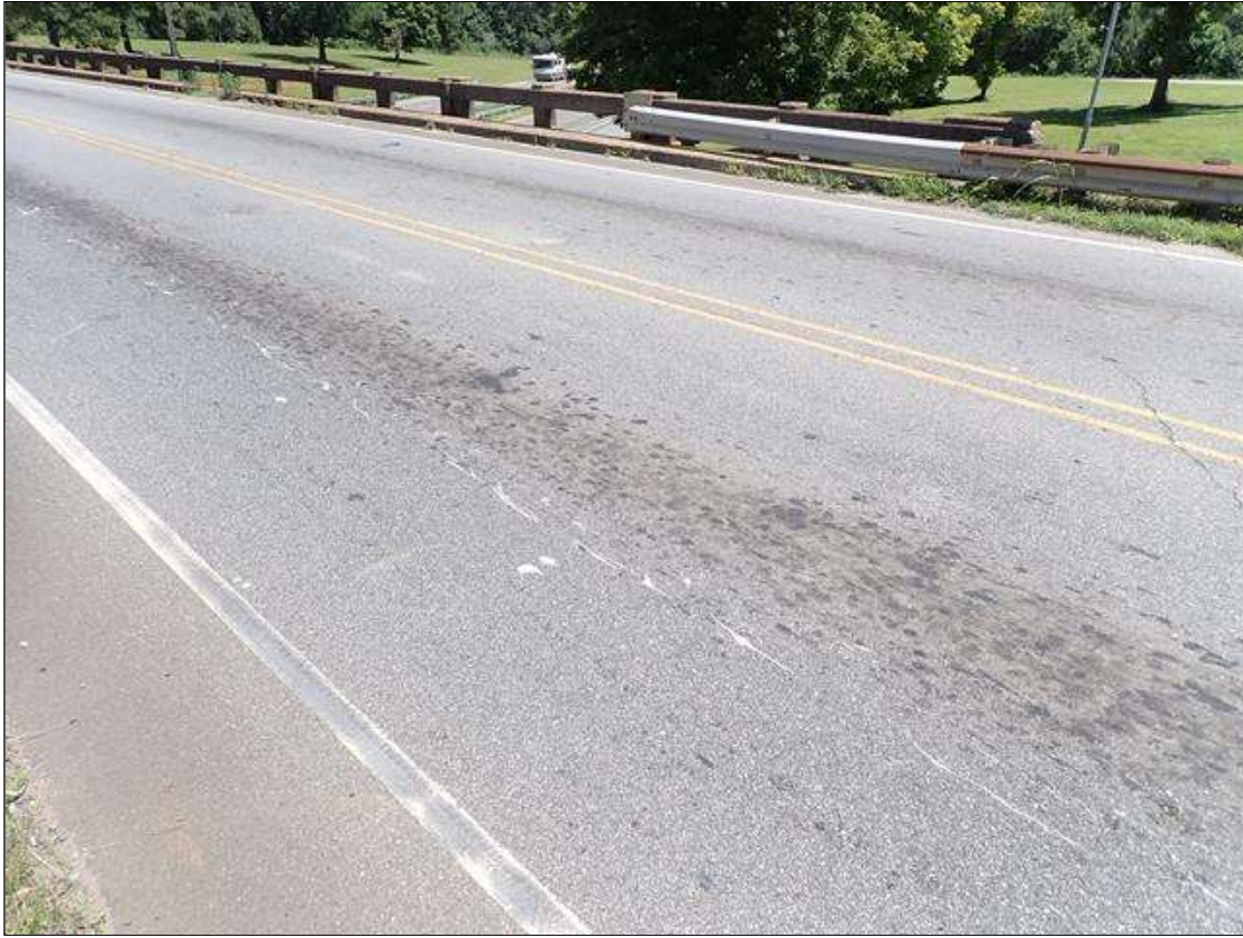
Span 1 Wearing Surface: (not found 2023) SPAN 1 WEARING SURFACE HAS SCATTERED PATCHED AREAS WITH SOME HAIRLINE CRACKS. PATCHES APPEAR TO BE SOUND. - NOT FOUND AT TIME OF INSPECTION. TDG 8/5/21
