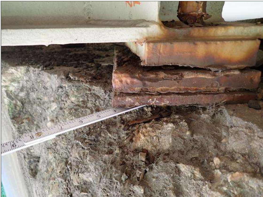
Span 3 Beam 2 - Near Bearing 2: [PAR] SPAN 3 BEAM 2 NEAR BEARING NORTHWEST CORNER HAS 5 INCH X 3 INCH X 4 INCH DEEP AREA OF BEARING LOSS. DUE TO BENT 2 CAP SPALLED AREA.
