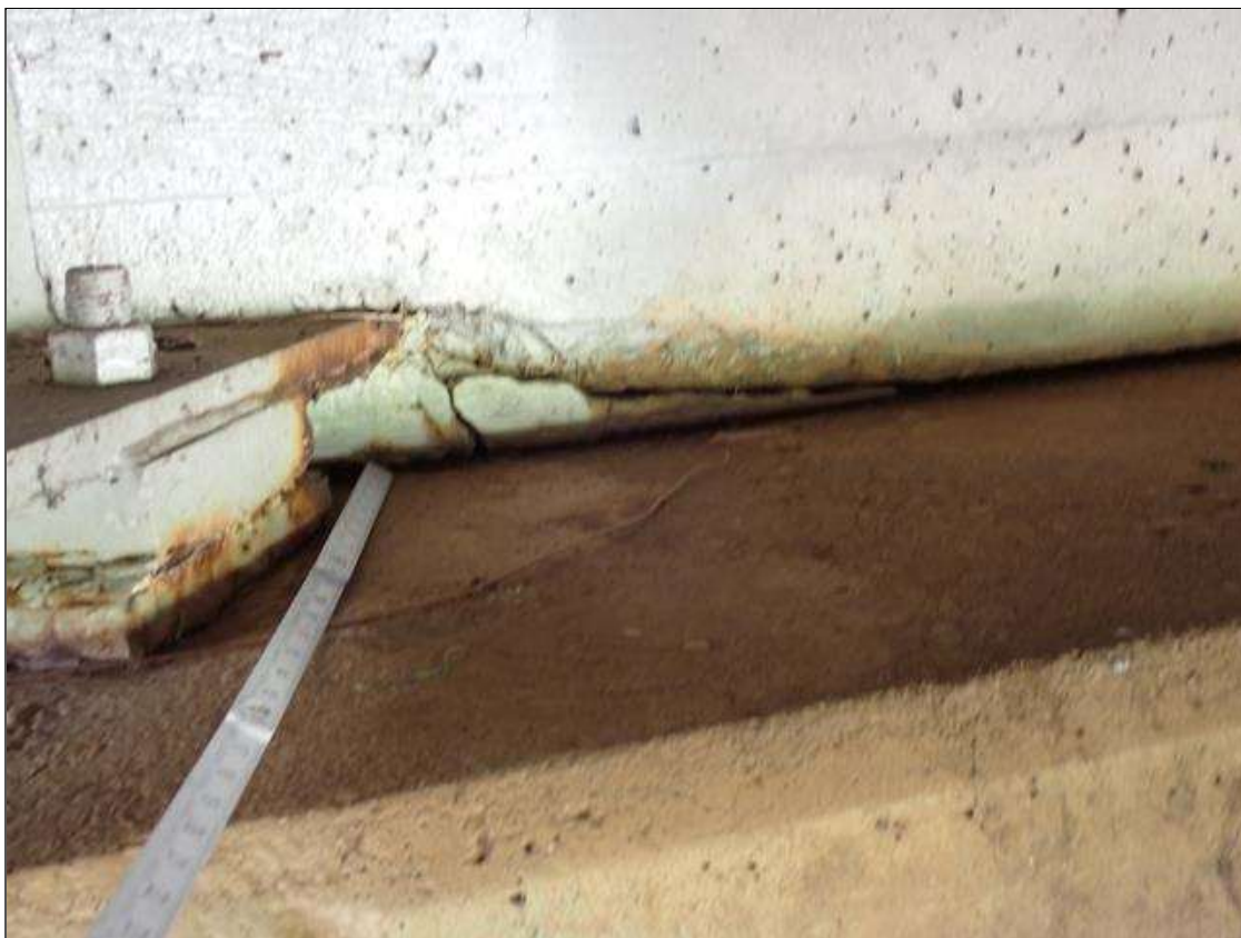
End Bent 2 Abutment: along the length of the abutment, at bottom flange penetrations, spall/delaminations (up to 1.5 foot x 3 inch x 1 inch) with cracks (up to 1/16 inch)
