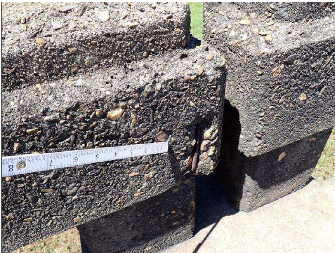
Span 4 Left Bridge Rail: 6th post from bent 3, spall (2 inch x 6 inch x 1 inch deep) with exposed rusted rebar
