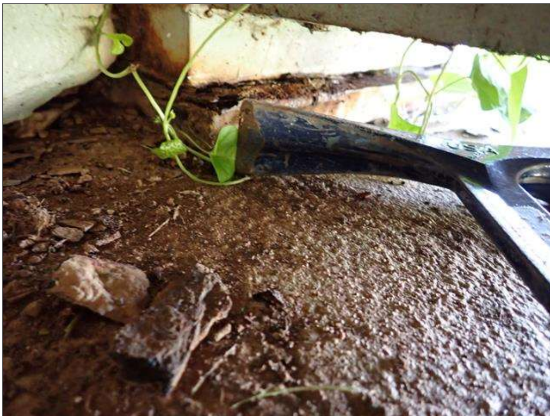
Span 1 Beam 1 - Near Bearing 1 - Protective System: surface rust/rust scale
