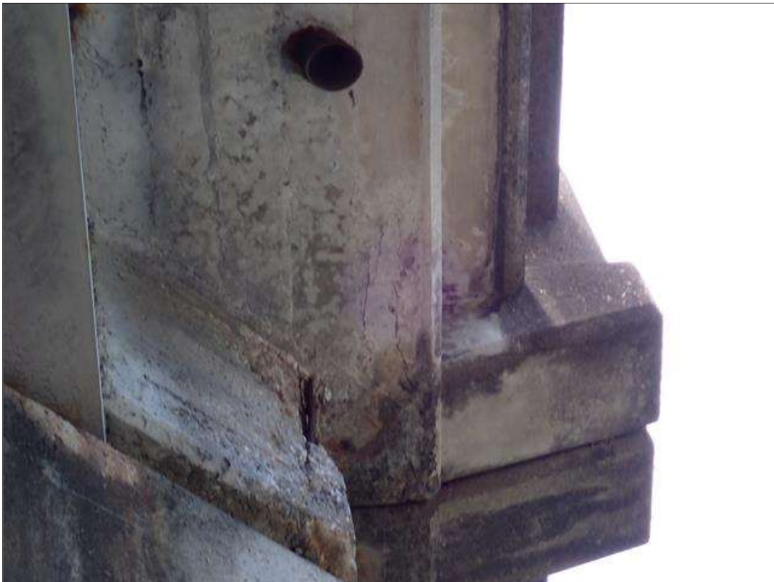
Span 3 Deck: AT BENT 3 UNDER RIGHT OVERHANG, DELAMINATION [28 INCHES X 12 INCHES ]
