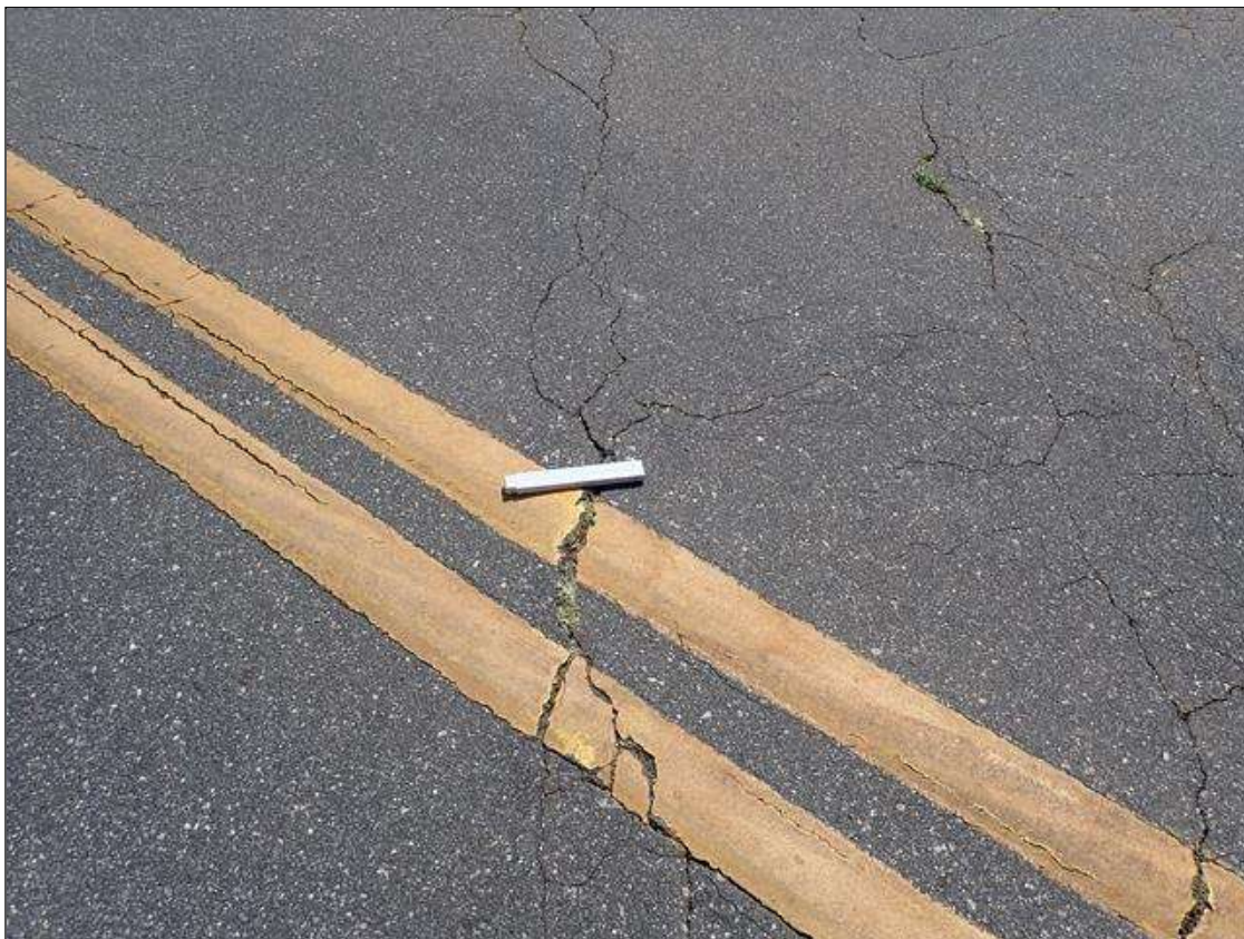
Span 1 Wearing Surface: 35 FEET X UP TO 1/4 INCHES TRANSVERSE CRACK OVER END BENT 1
