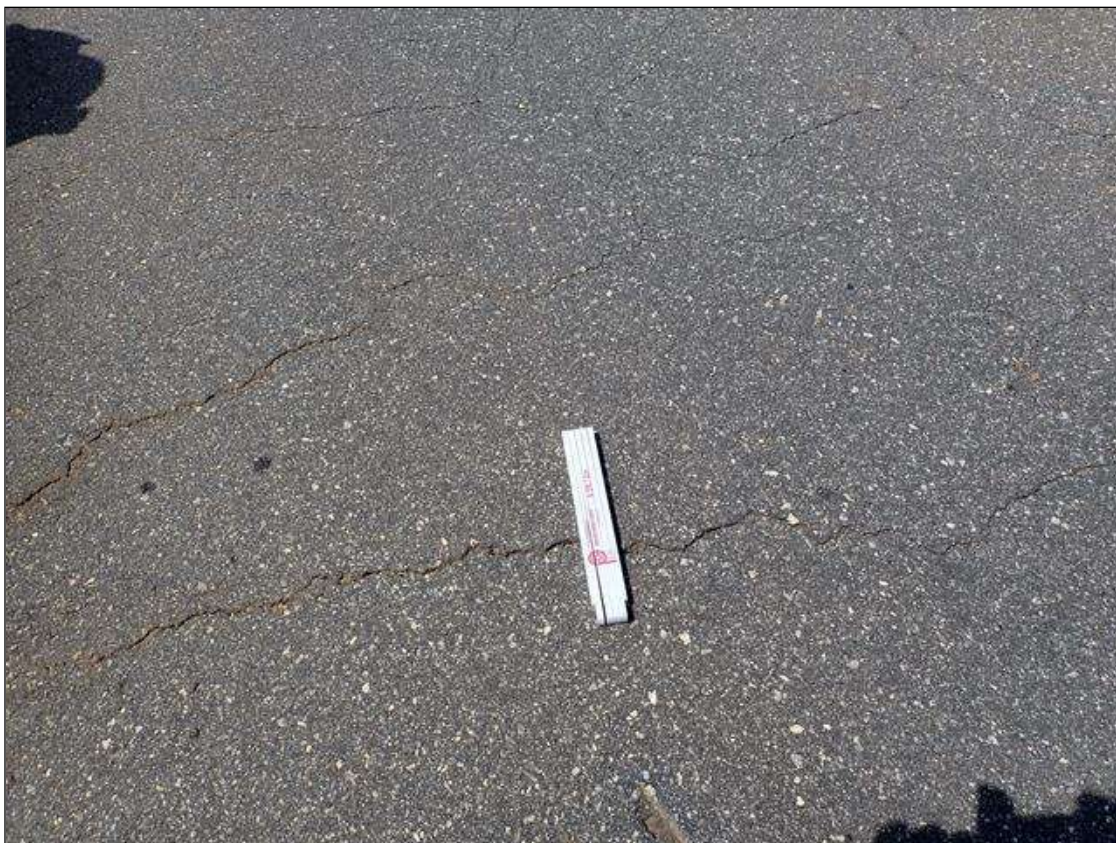
Span 4 Wearing Surface: ASPHALT WEARING SURFACE HAS SCATTERED MAP CRACKING [UP TO 1/8 INCHES ] AT RANDOM THROUGHOUT
