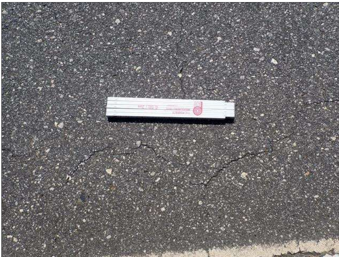
Span 1 Wearing Surface: ASPHALT WEARING SURFACE HAS SCATTERED MAP CRACKING UP TO 1/32 INCHES THROUGH OUT
