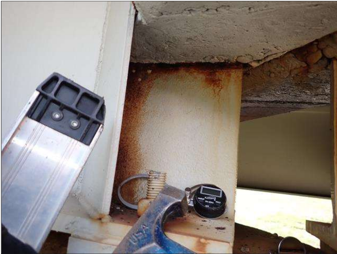
Span 2 Beam 4: at bent 2, web adjacent to end diaphragm, corrosion with section loss (9/16 inch average remaining x 10 inch x 1 inch)
