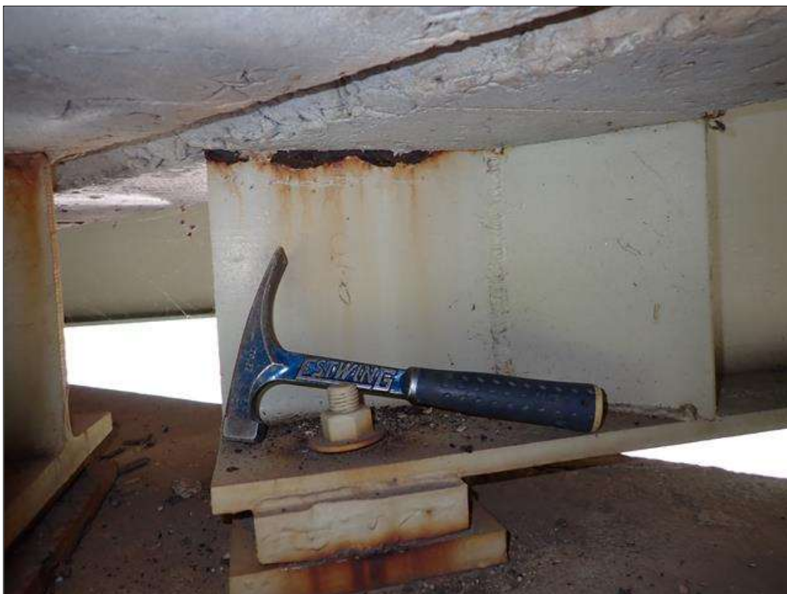
Span 3 Beam 2: at bent 2, web adjacent to end diaphragm, rust scale (10 inch)
