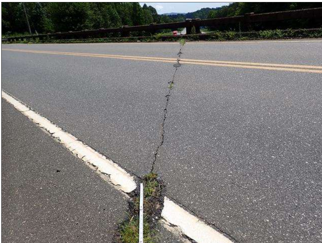
Span 3 Wearing Surface: 35 FEET X UP TO 1/8 INCHES TRANSVERSE CRACK WITH EDGE SPALLS UP TO 2 FOOT X 4 INCH X 1 INCH DEEP WITH VEGETATION GROWTH OVER BENT 2
