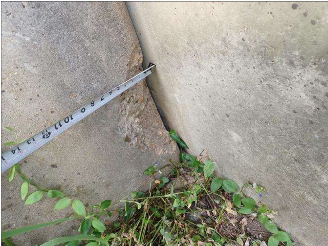
Bent 1 Pile 3: BOTTOM EAST FACE OF COLUMN 3 HAS A SPALL AREA AT GROUND LINE 7 INCHES X 17 INCHES X 3.5 INCHES .
