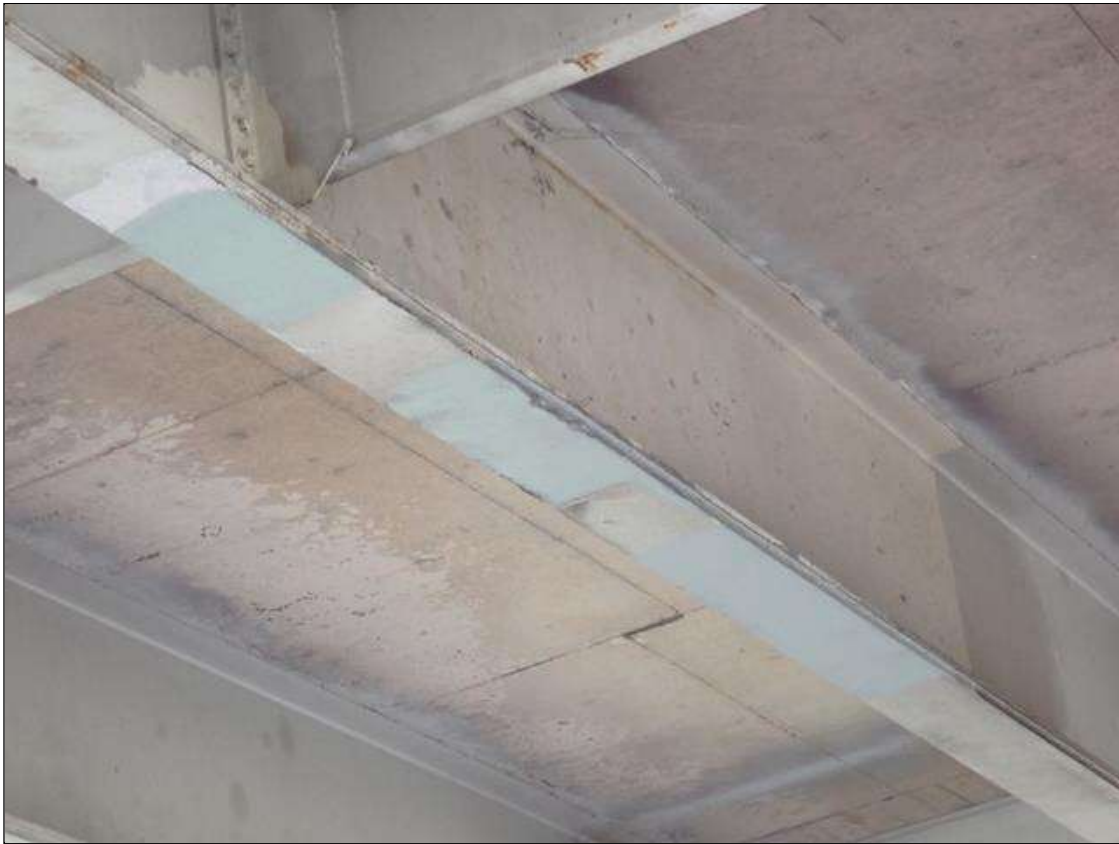
Span 2 Beam 3: 2023 new repair, previously noted as: SUPPLEMENTAL INSPECTION 2021: POINT OF IMPACT ON BEAM 3 26 FEET 1 INCHES FROM FACE OF BENT 1. A INDENTION IN COVER PLATE THREE INCHES X 1/2 INCHES AND A 2 INCHES X 1/2 INCHES IN THE IMPACT AREA.
