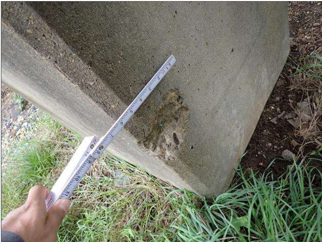
Bent 2 Pile 1: 5 INCHES X 5 INCHES X 1 INCHES SPALL ON SOUTH WEST CORNER 18 INCHES ABOVE THE GROUND.
