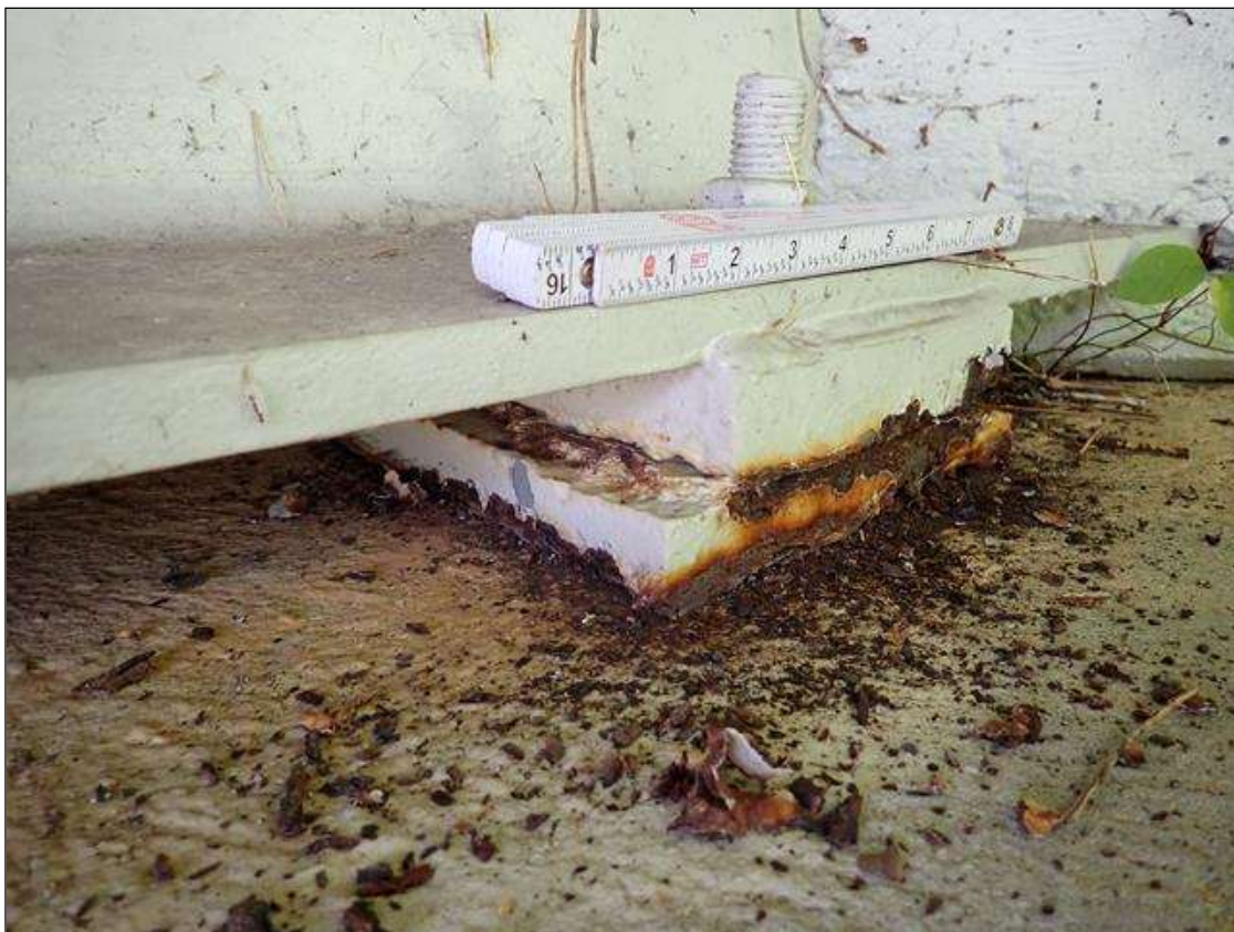
Span 1 Near Bearing 1: corrosion with section loss (up to 1/8 inch loss)
