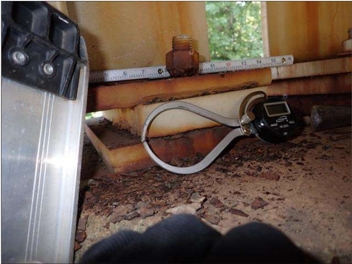
Span 2 Near Bearing 4: surface rust/rust scale
