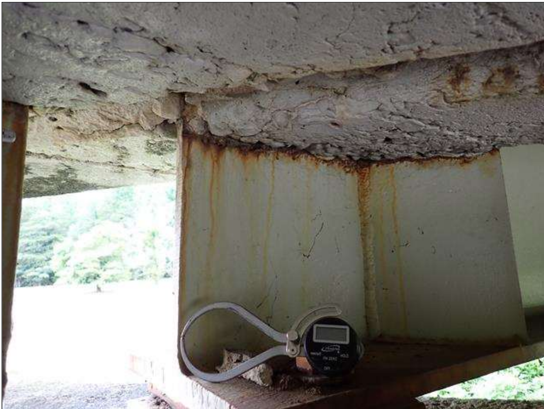
Span 4 Beam 1: at bent 3, web adjacent to end diaphragm, corrosion with section loss (9/16 inch average remaining x 10 inch x 1 inch)
