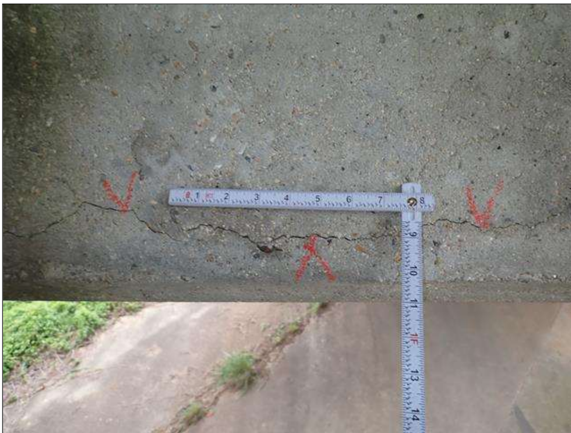
Bent 1 Cap 1: BOTH FACES OF CAP, MULTIPLE HORIZONTAL AND VERTICAL CRACKS [UP TO 7 FEET X 1/16 INCHES ]
