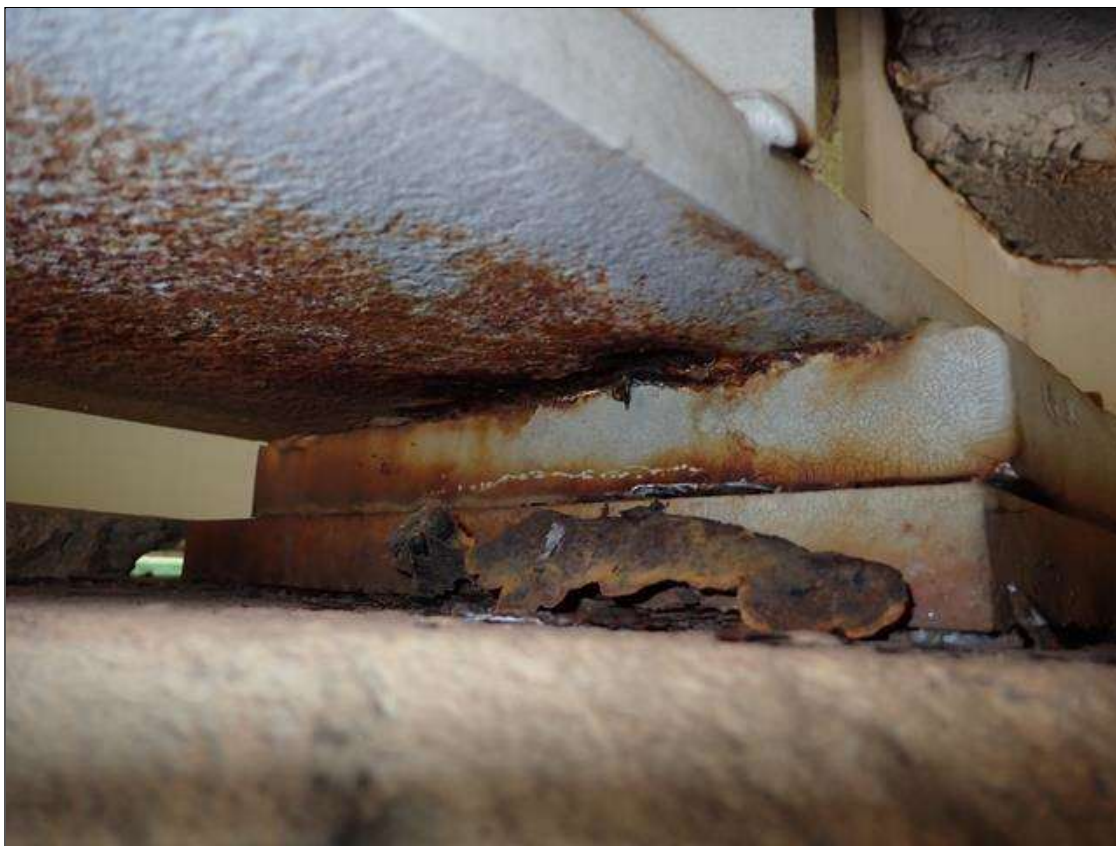
Span 2 Beam 3: at bent 1, web adjacent to end diaphragm and bottom flange, rust scale (13 inch)
