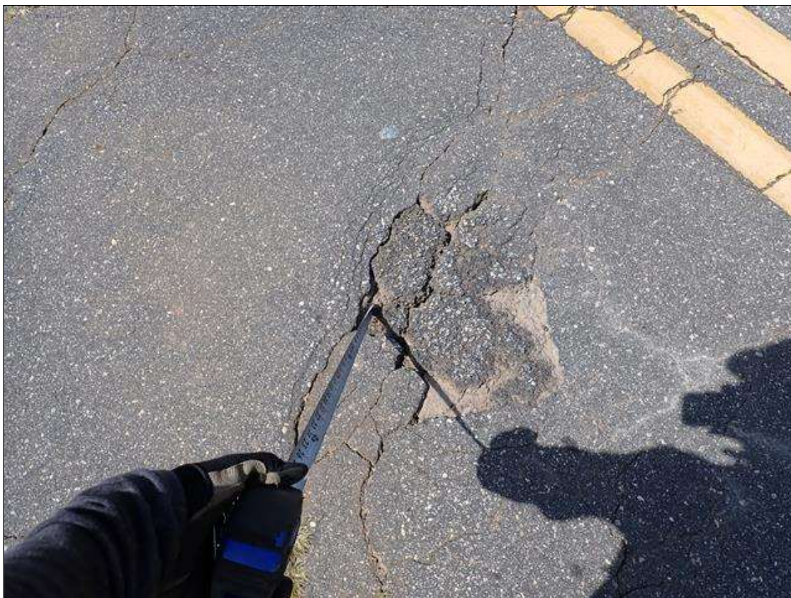
(PAR) north approach asphalt wearing surface, northbound lane near end bent 2, broken asphalt (3 foot x 2 foot x 1.5 inch deep)
