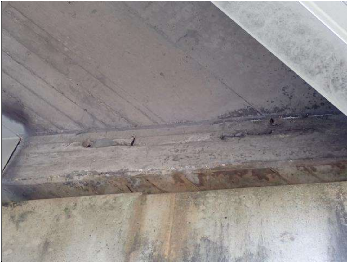
Span 3 Beam 4: BAY 3 DIAPHRAGM OVER BENT 3, SPALL/DELAMINATION [2] [UP TO 6 INCHES X 3 INCHES X UP TO 3/4 INCHES DEEP] WITH EXPOSED RUSTED REINFORCING
