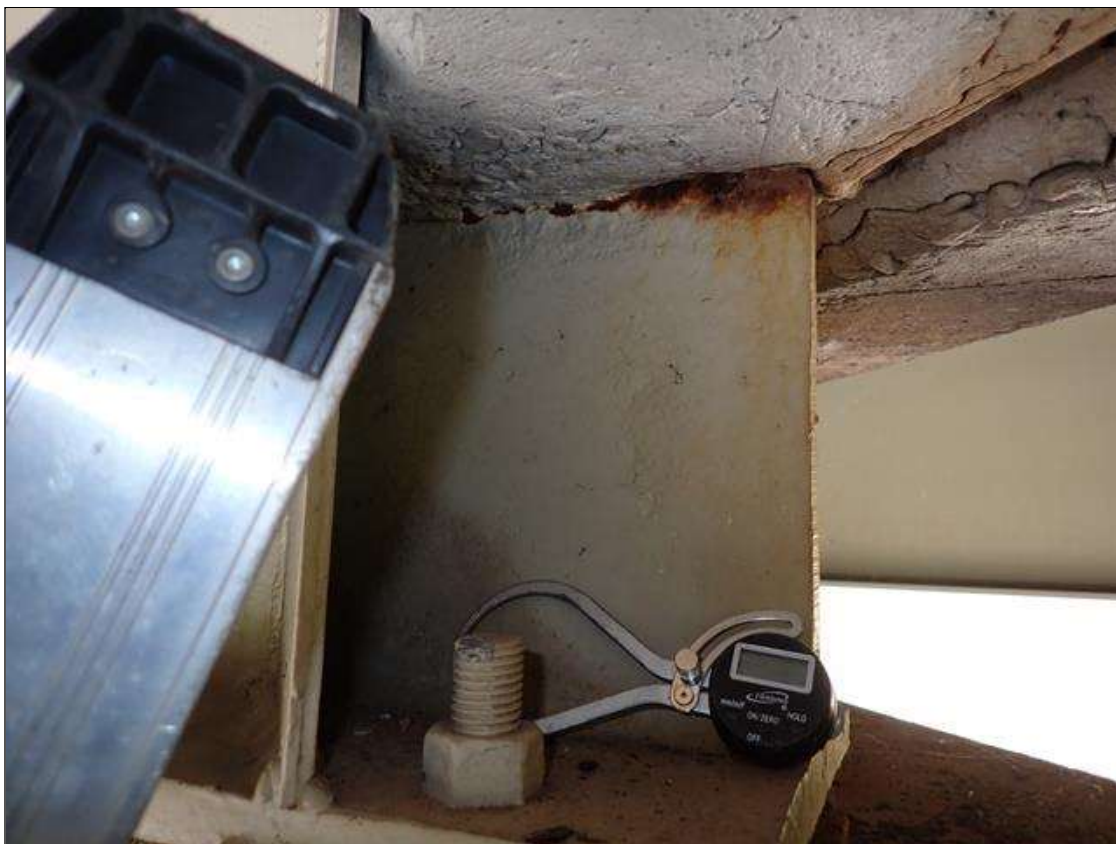
Span 2 Beam 3: at bent 2, web adjacent to end diaphragm, corrosion with section loss (9/16 inch average remaining x 10 inch x 1 inch)
