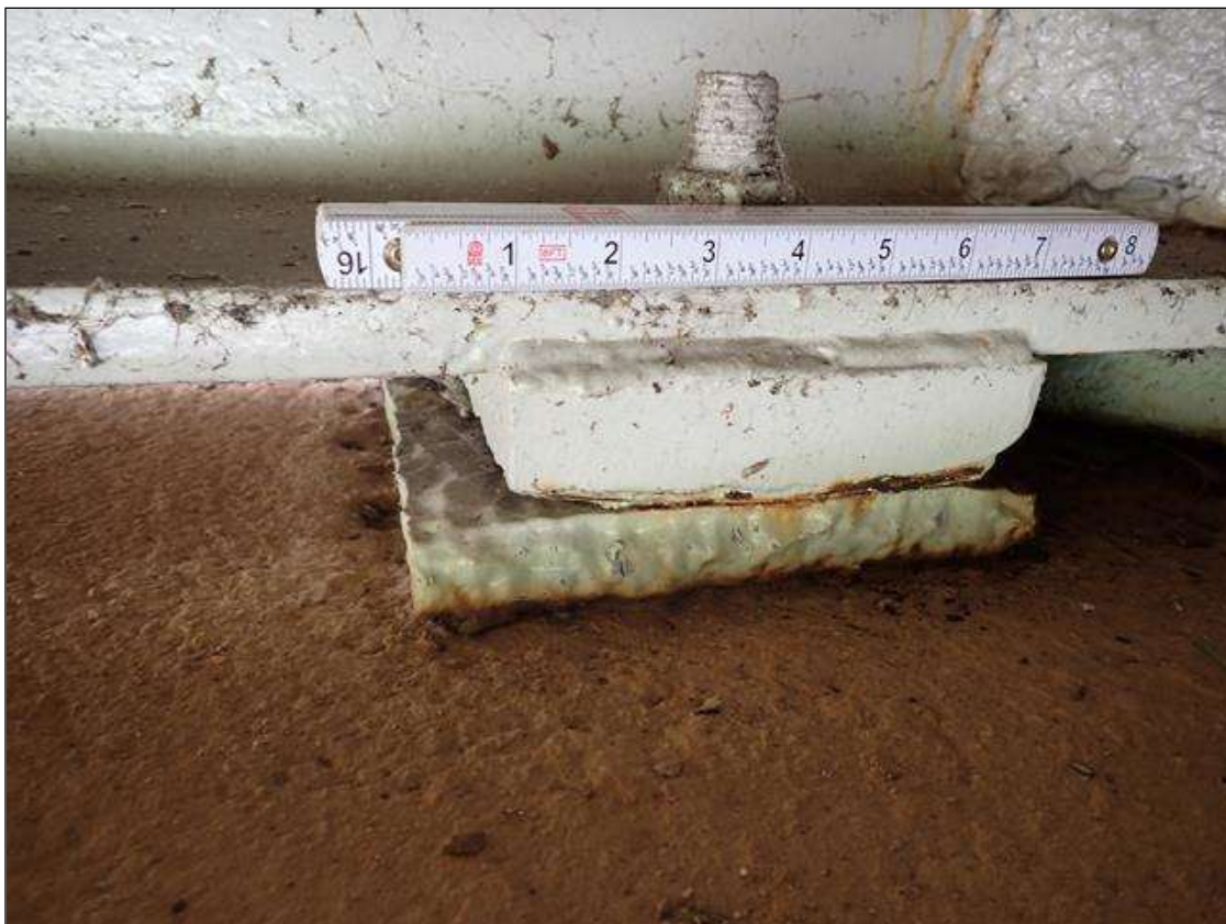
Span 1 Beam 4 - Near Bearing 4: corrosion with section loss (up to 1/8 inch loss)
