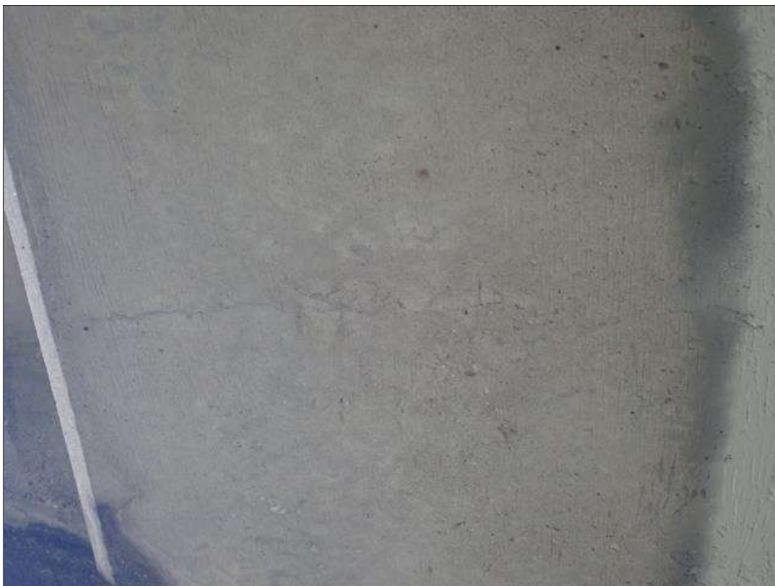
Span 1 Deck: ALONG BOTH OVERHANGS, TRANSVERSE CRACKS UP TO 1/32 INCH X FULL WIDTH
