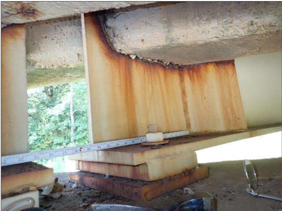
Span 1 Beam 4: at bent 1, web adjacent to end diaphragm, rust scale (13 inch)
