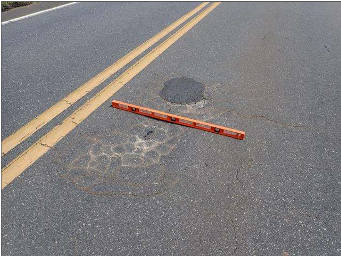
Span 1 Wearing Surface: ASPHALT WEARING SURFACE IS BROKEN UP/PARTIALLY PATCH AND DEPRESS IN A FEET X 6 FEET X 1 INCH DEEP AREA 12 FEET FROM END BENT 1 AND 9 FEET FROM RIGHT CURB.
