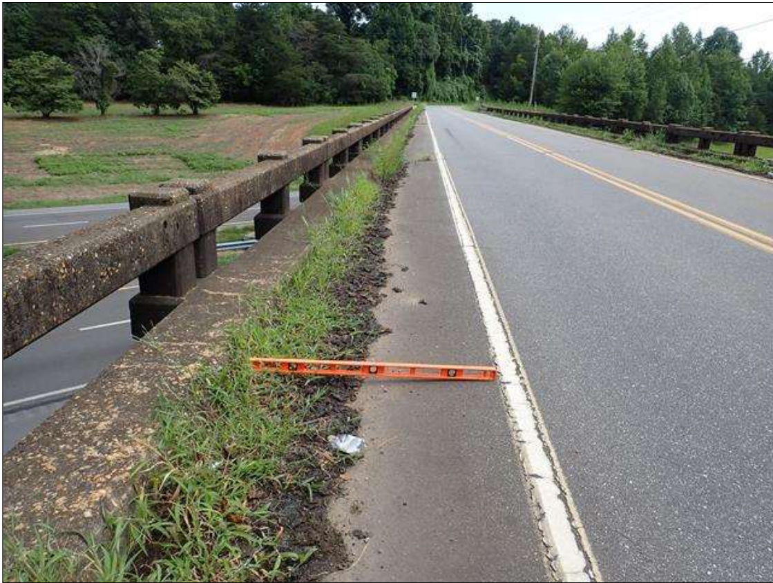
along both curblines, debris accumulation (up to 2 foot wide x full length); fully obstructing drainage
