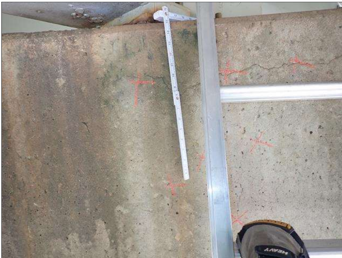
Bent 2 Cap 1: ALONG ALL FACES OF CAP, SCATTERED MAP CRACKING UP TO 1/64 INCHES AT RANDOM
