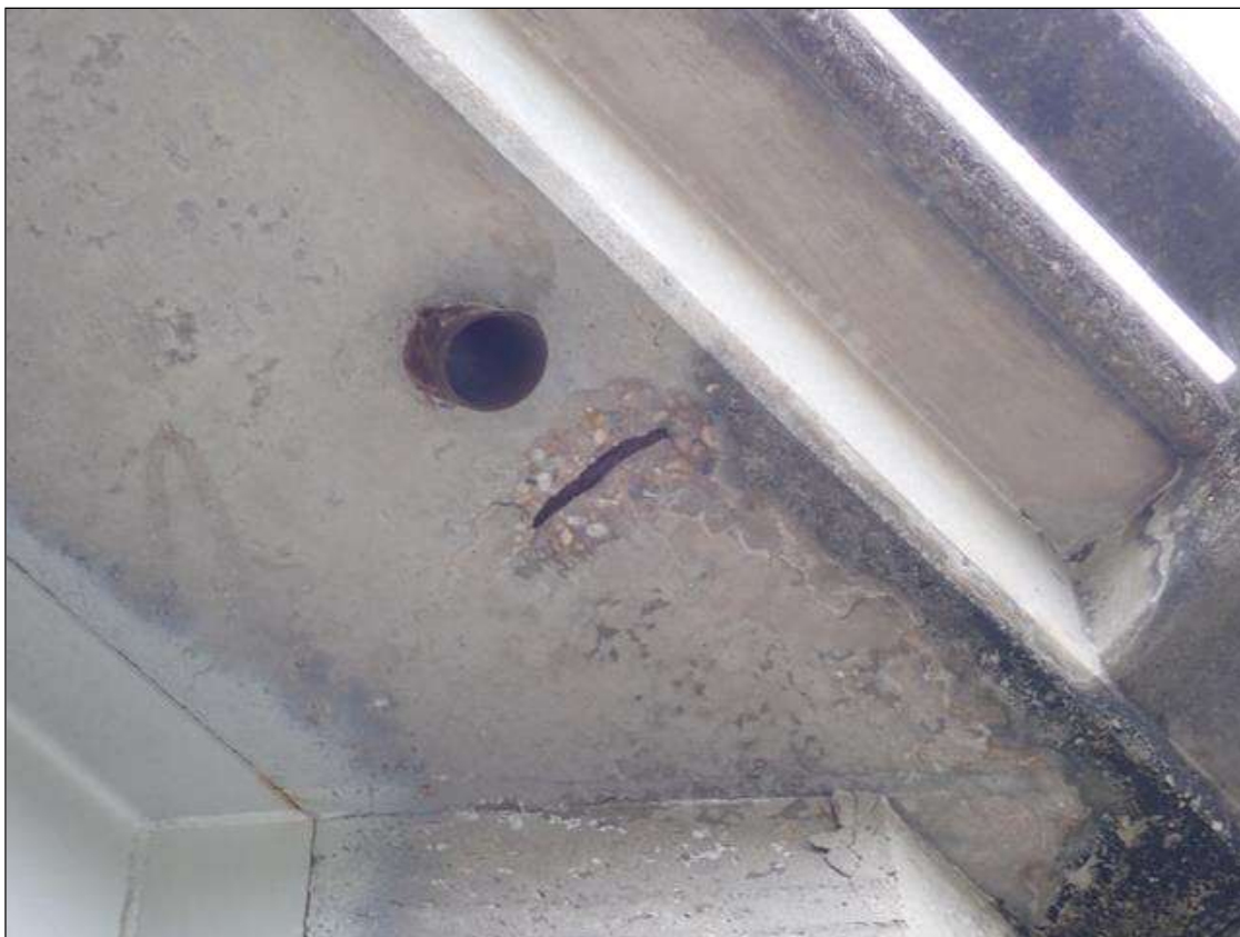
Span 2 Deck: (PAR) west overhang over bent 1, spall (18 inch x 6 inch x 1/2 inch deep) with exposed rusted rebar
