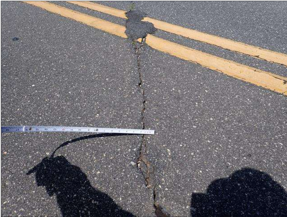
Span 2 Wearing Surface: 35 FEET X UP TO 1/8 INCHES TRANSVERSE CRACK OVER BENT 1 WITH EDGE SPALLS UP TO 3 INCH X 1 INCH DEEP
