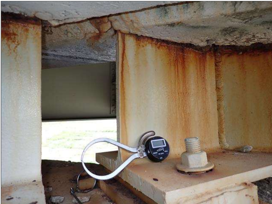
Span 3 Beam 4: at bent 2, web adjacent to end diaphragm, corrosion with section loss (9/16 inch average remaining x 10 inch x 1 inch)
