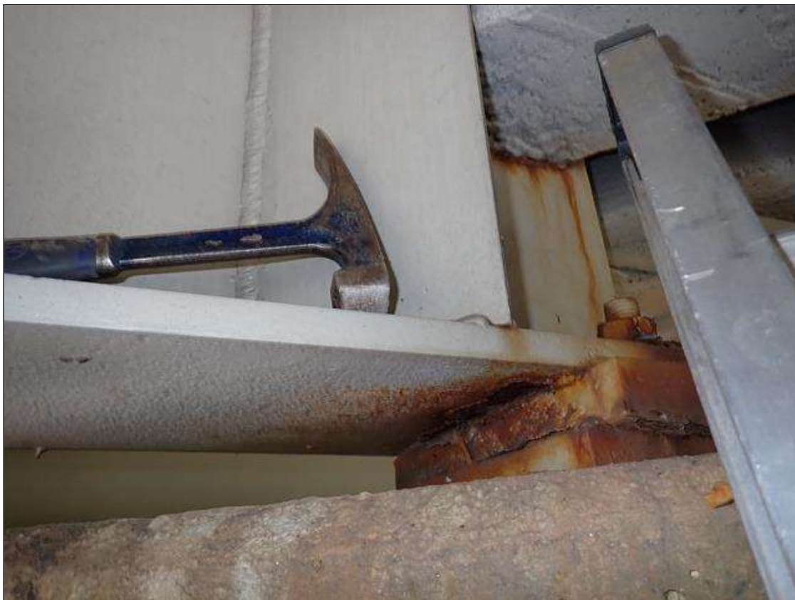
Span 2 Beam 2: at bent 1, web adjacent to end diaphragm and bottom flange, rust scale (13 inch)
