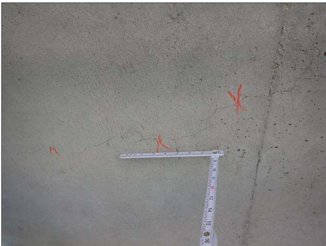
Span 1 Deck: BOTTOM OF DECK HAS SCATTERED AREAS OF TRANSVERSE CRACKS UP TO 1/32 INCHES X FULL WIDTH SOME WITH EFFLORESCENCE AT RANDOM THROUGHOUT
