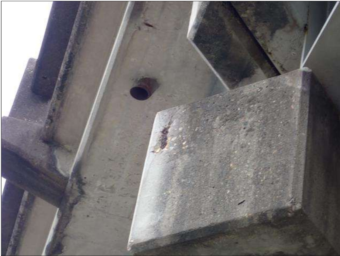
Bent 2 Cap 1: WEST END OF CAP HAS A SURFACE SPALL AND DELAMINATED AREA 4 INCHES X 10 INCHES X 1/2 INCHES WITH EXPOSED RUSTED REINFORCING [NO LOSS]
