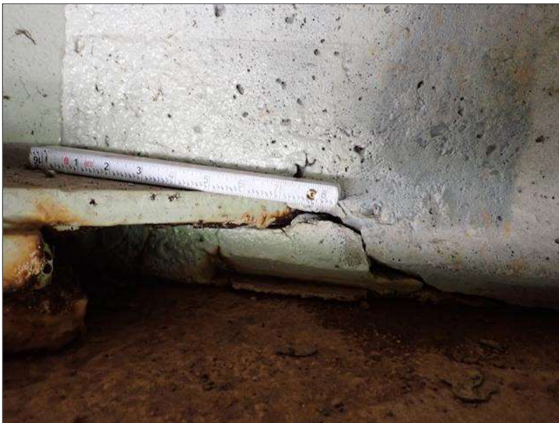
End Bent 2 Abutment: AT ALL BEAM PENETRATIONS, MULTIPLE SPALLS/DELAMINATIONS [UP TO 10 INCHES X 1 INCHES X 1 INCHES DEEP]
