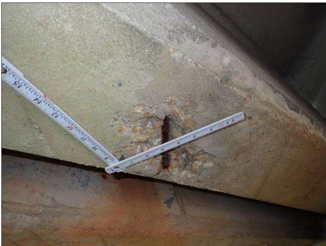
Span 2 Beam 2: 8 INCH X UP TO 5 INCH X 1/2 INCH DEEP SPALL WITH EXPOSED REINFORCING BOTTOM FACE OF BENT 1 DIAPHRAGM IN BAY 2
