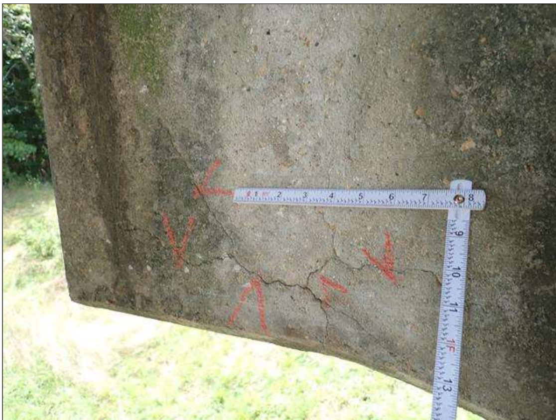
Bent 1 Cap 1: MAP CRACKS (UP TO 1/32 INCH X 2 FOOT X UP TO FULL HEIGHT) NORTHEAST BOTTOM CORNER.
