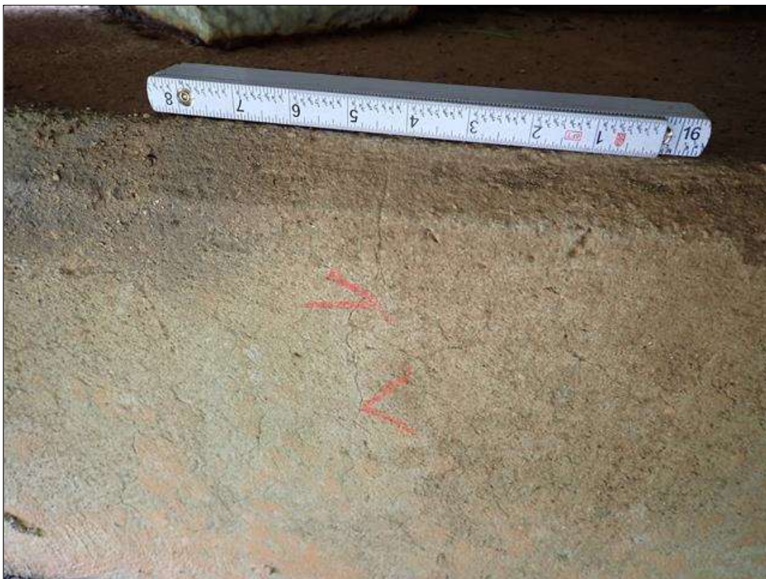
End Bent 1 Cap 1: ALONG LENGTH, MULTIPLE VERTICAL CRACKS [UP TO FULL HEIGHT X 1/64 INCHES ]
