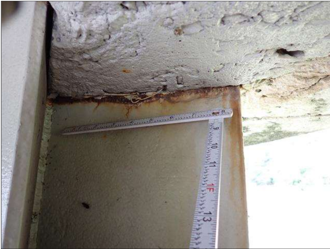
Span 3 Beam 1: at bent 3, web adjacent to end diaphragm, corrosion with section loss (9/16 inch average remaining x 10 inch x 1 inch)
