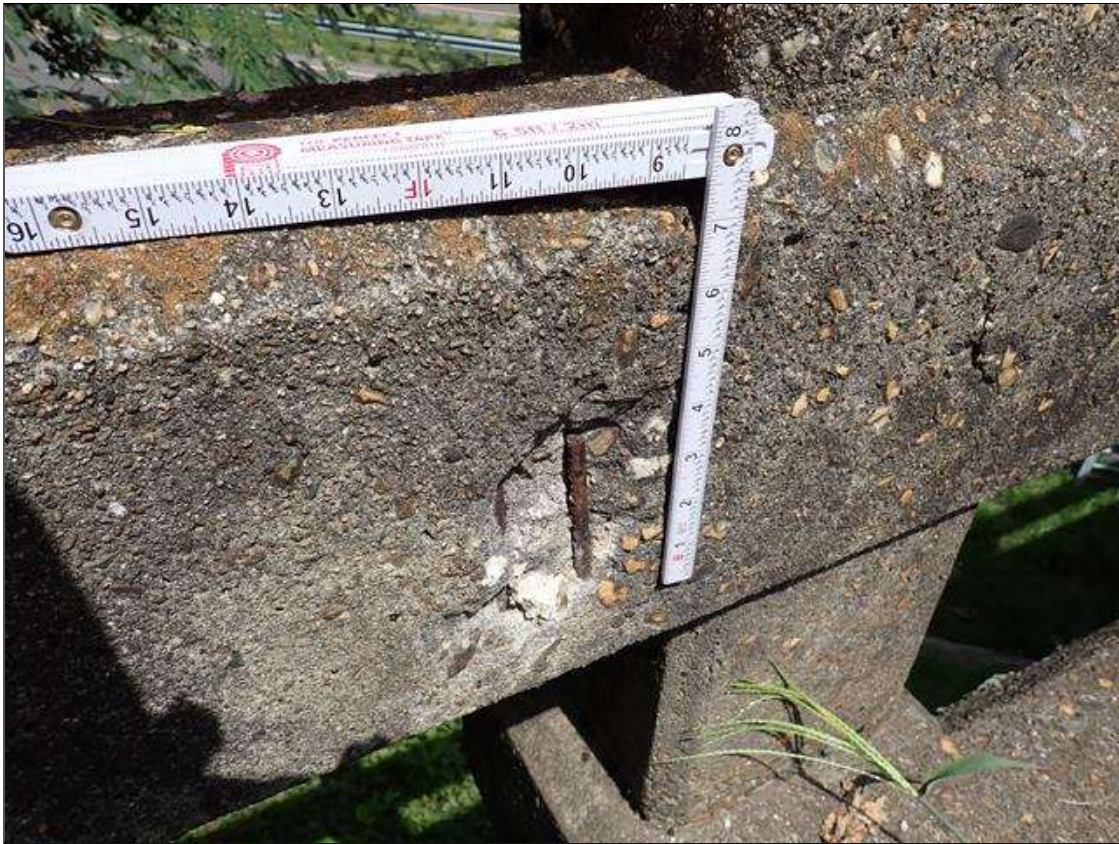
Span 1 Left Bridge Rail: (4) UP TO 5 INCHES DIAMETER X 1/2 INCHES SPALLS WITH EXPOSED REINFORCING 20 FEET FROM END BENT 1 NO SECTION LOSS
