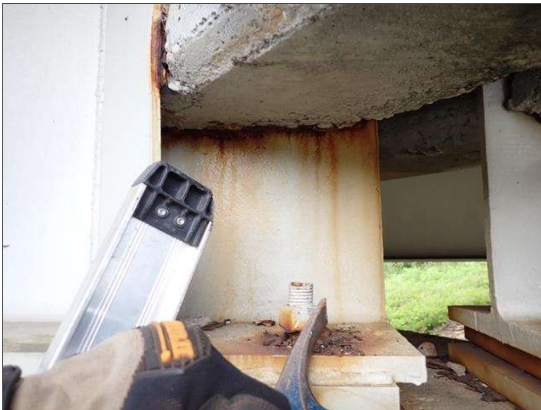
Span 2 Beam 1: at bent 1, web adjacent to end diaphragm and bottom flange, rust scale (13 inch)
