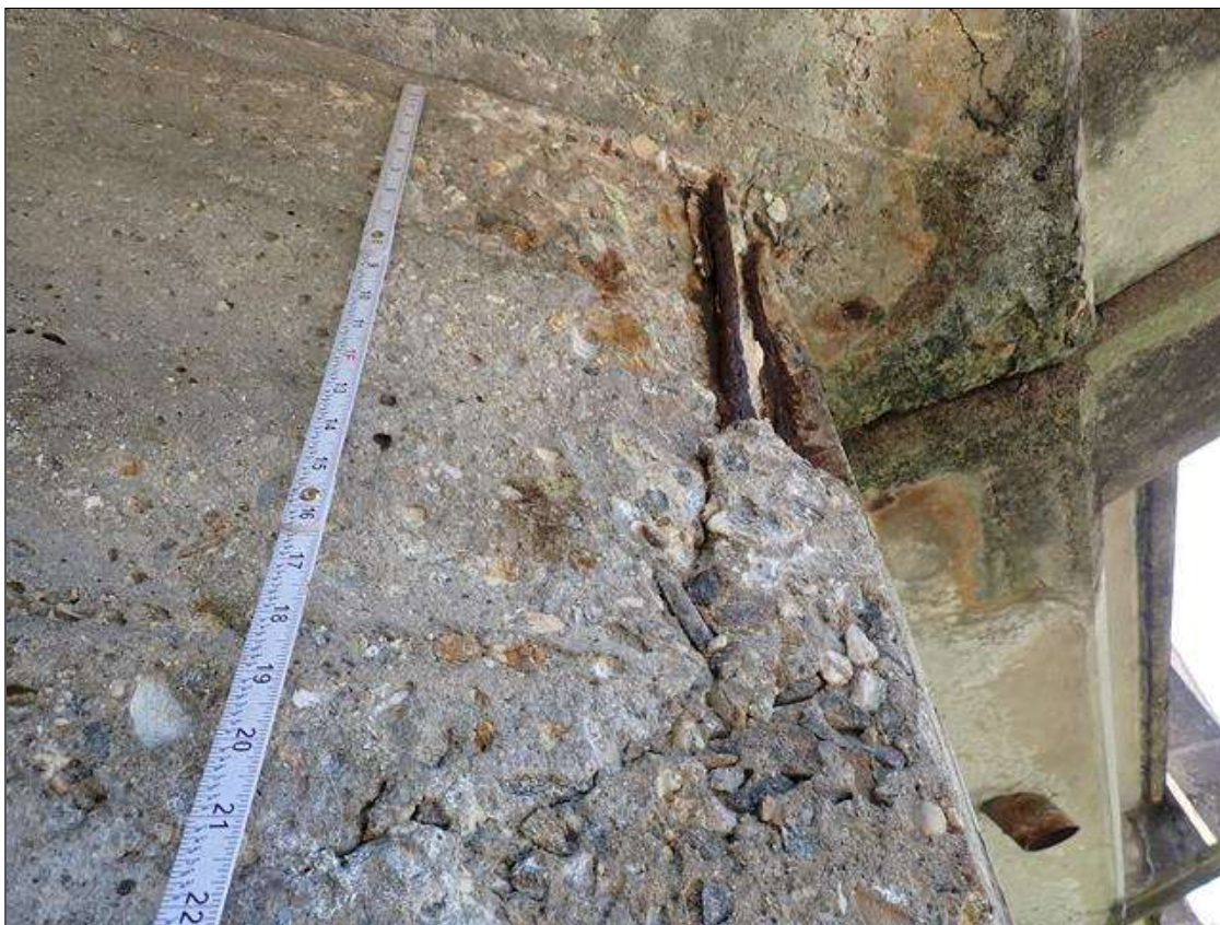
Span 3 Beam 4: (PAR) DIAPHRAGM OVER BENT 3 UNDER RIGHT OVERHANG, DELAMINATION/SPALL [FULL HEIGHT X 2 FOOT X 2 INCHES DEEP] WITH TWO [2] EXPOSED RUSTED REINFORCING WITH APPROXIMATELY 25 PERCENT LOSS
