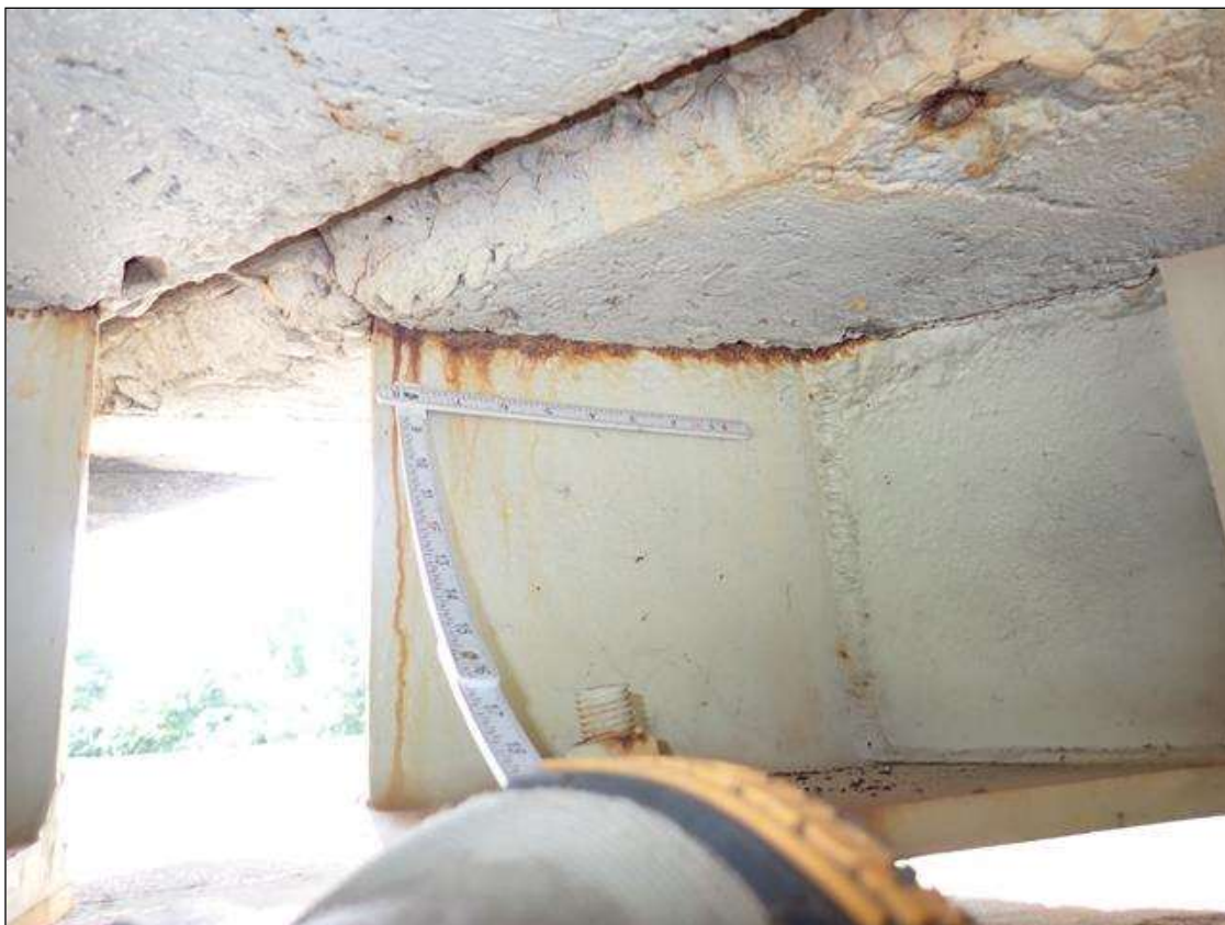
Span 3 Beam 1: at bent 2, web adjacent to end diaphragm, corrosion with section loss (9/16 inch average remaining x 10 inch x 1 inch)
