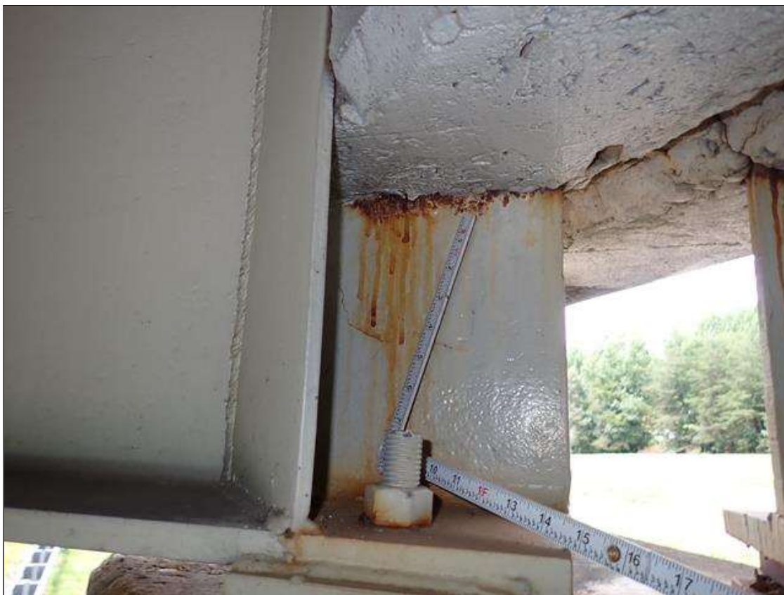
Span 2 Beam 1: at bent 2, web adjacent to end diaphragm, rust scale (10 inch)
