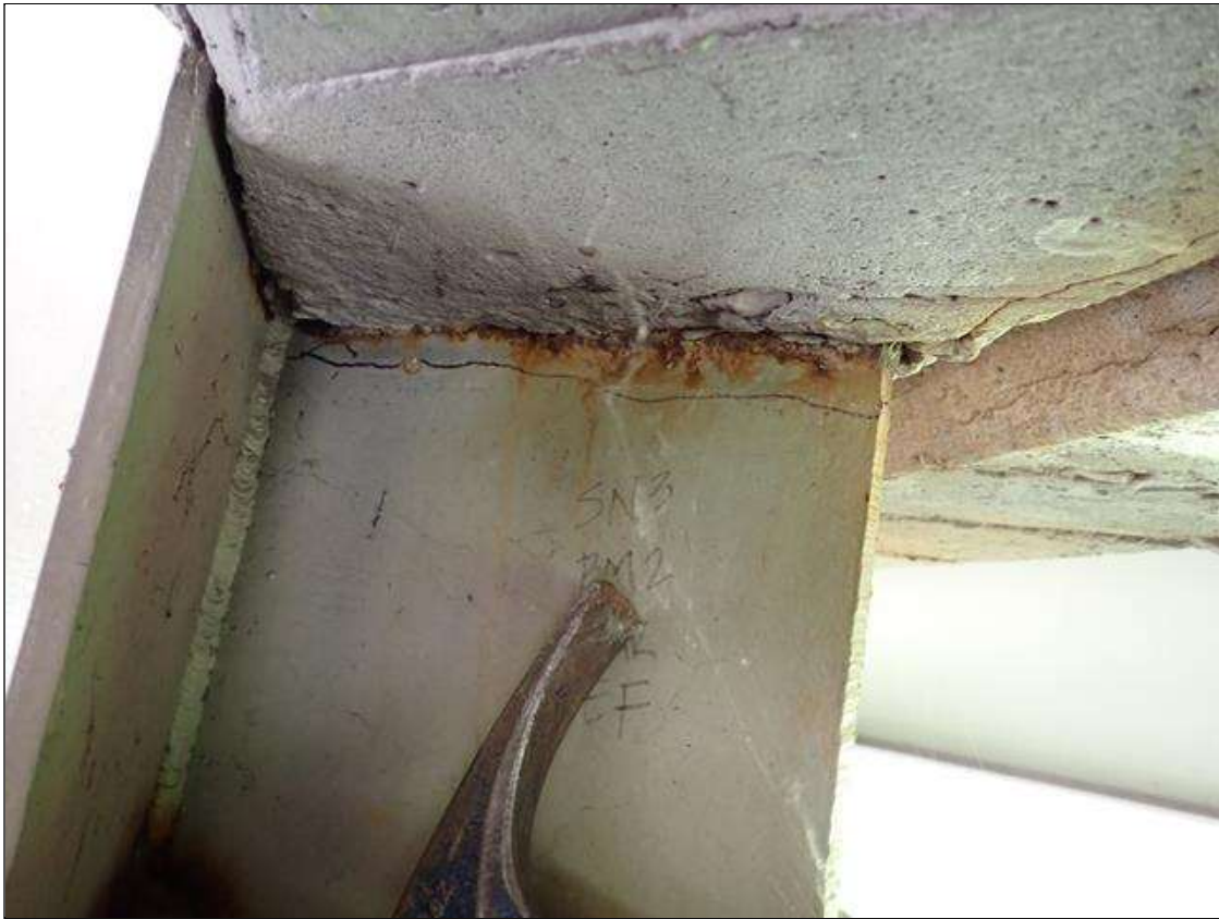
Span 3 Beam 2: at bent 3, web adjacent to end diaphragm, corrosion with section loss (9/16 inch average remaining x 10 inch x 1 inch)
