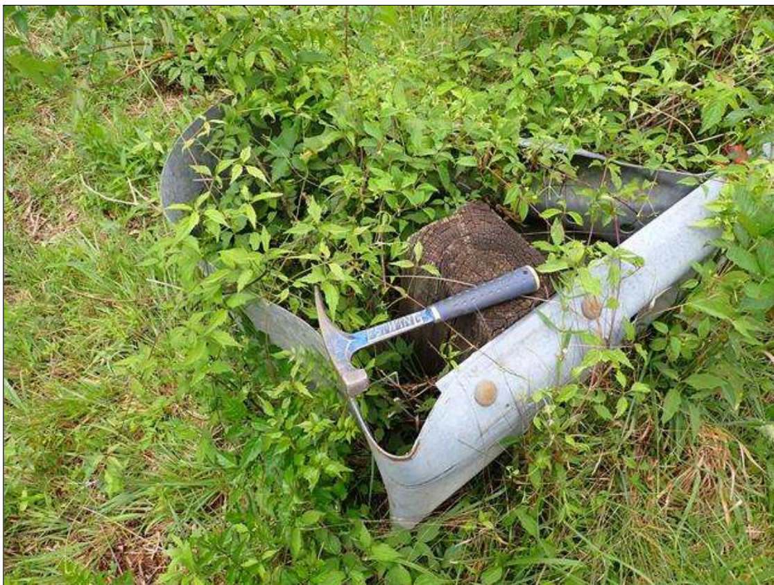
(PAR) northeast guardrail termination, impact damage
