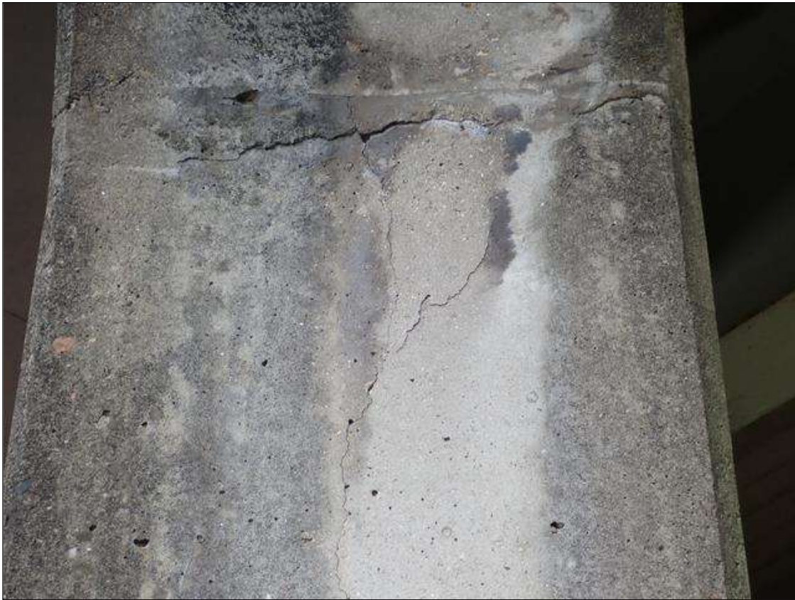
Bent 1 Pile 1: WEST FACE AT CAP, VERTICAL CRACK [4 FEET X UP TO 1/32 INCHES ] WITH ADJACENT DELAMINATION [10 INCHES X 6 INCHES ]
