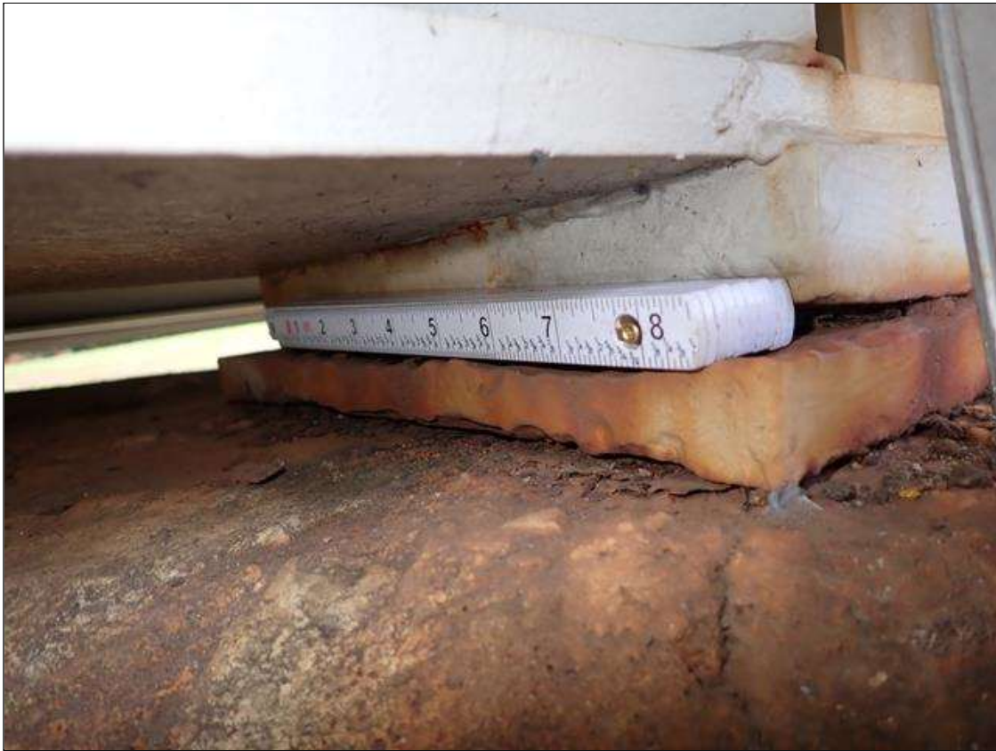
Span 2 Far Bearing 4: corrosion with section loss (up to 1/8 inch loss)
