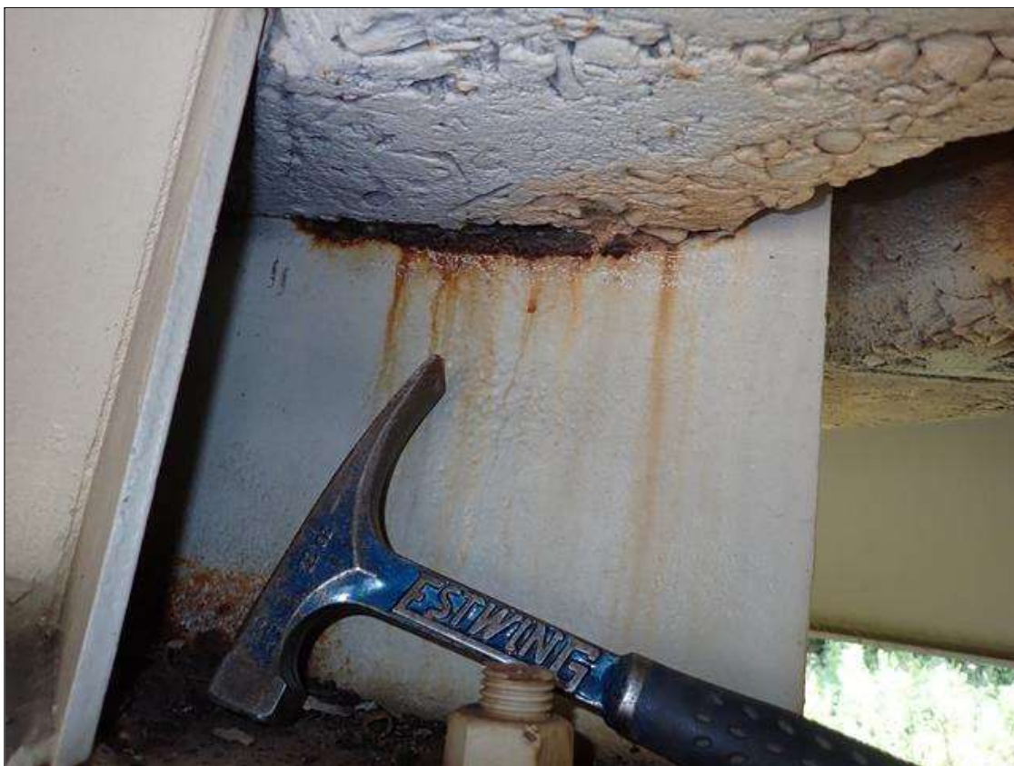
Span 2 Beam 3: at bent 1, web adjacent to end diaphragm and bottom flange, rust scale (13 inch)
