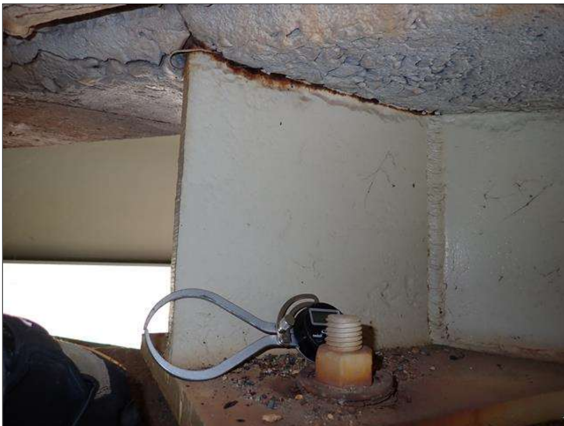
Span 3 Beam 3: at bent 2, web adjacent to end diaphragm, corrosion with section loss (9/16 inch average remaining x 10 inch x 1 inch)
