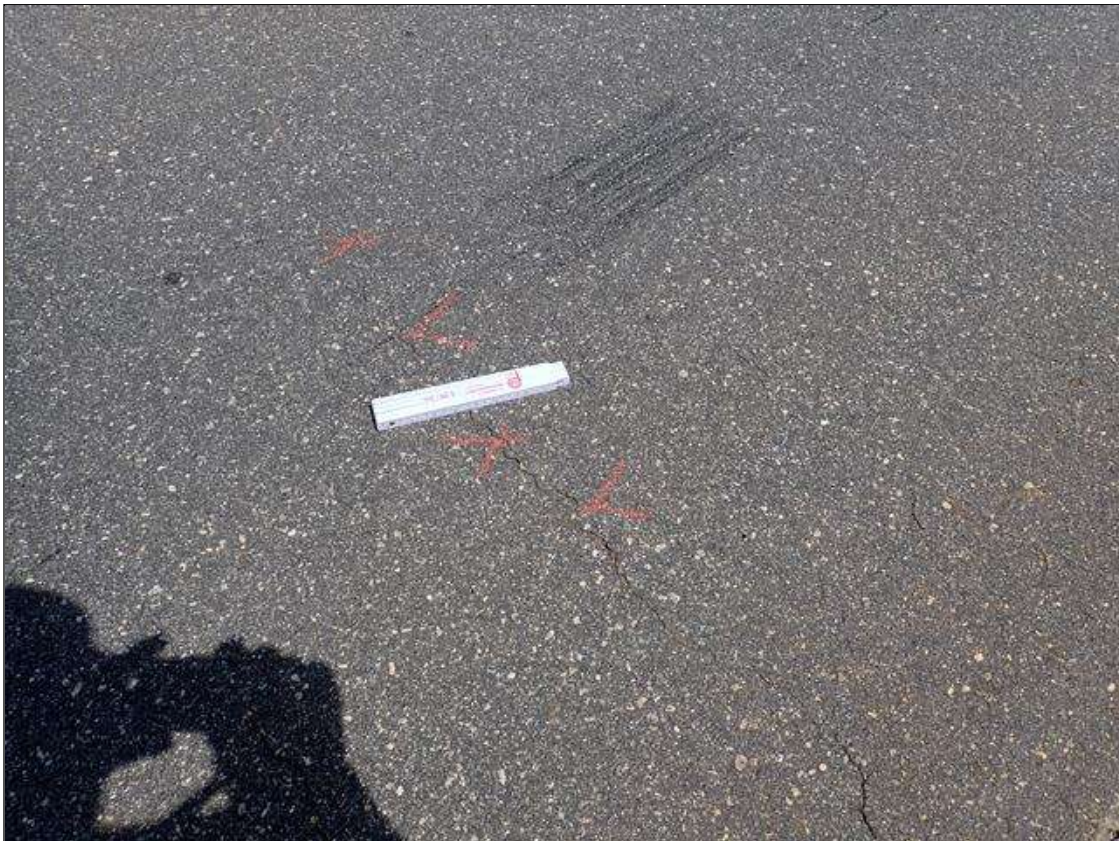
Span 2 Wearing Surface: TRANSVERSE CRACKS UP TO 1/16 FEET INCH X 12 FOOT AND MAP CRACKS UP TO 1/32 AT RANDOM THROUGHOUT
