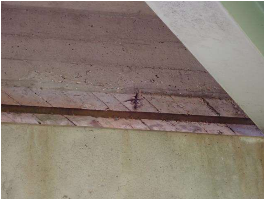
Span 4 Beam 2: BAY 2 END DIAPHRAGM OVER BENT 3, SPALL [8 INCHES X 6 INCHES X 1/2 INCHES DEEP] WITH EXPOSED RUSTED REINFORCING
