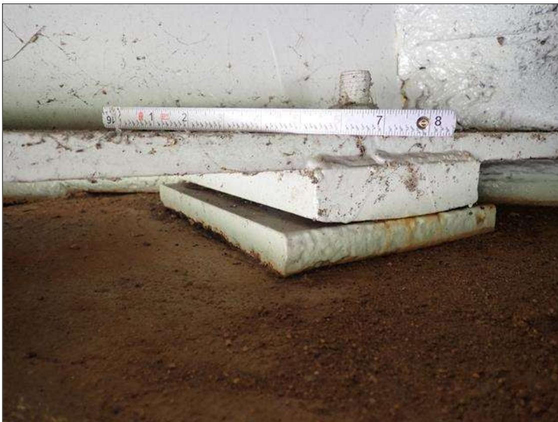
Span 1 Near Bearing 3: painted over pitting (up to 1/16 inch deep)
