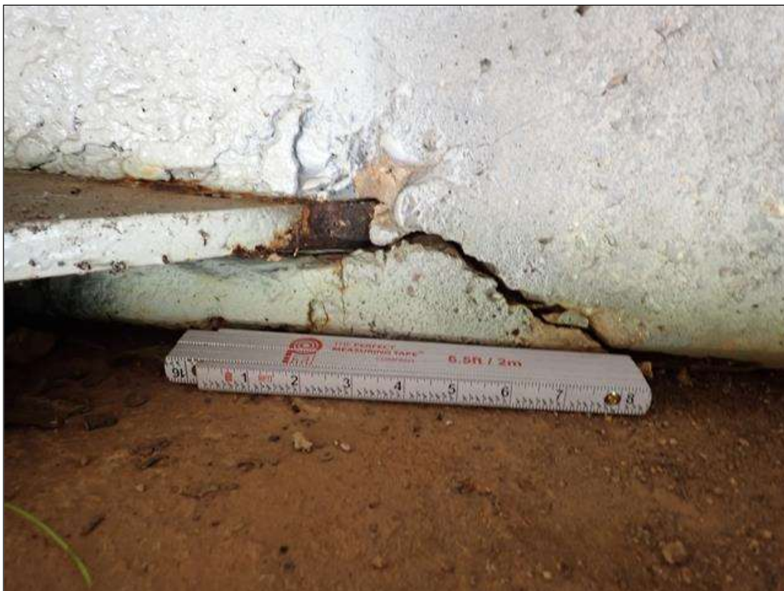
End Bent 1 Abutment: AT ALL BEAM PENETRATIONS, MULTIPLE SPALLS/DELAMINATIONS [UP TO 9 INCHES X 5 INCHES X 1 INCHES DEEP]
