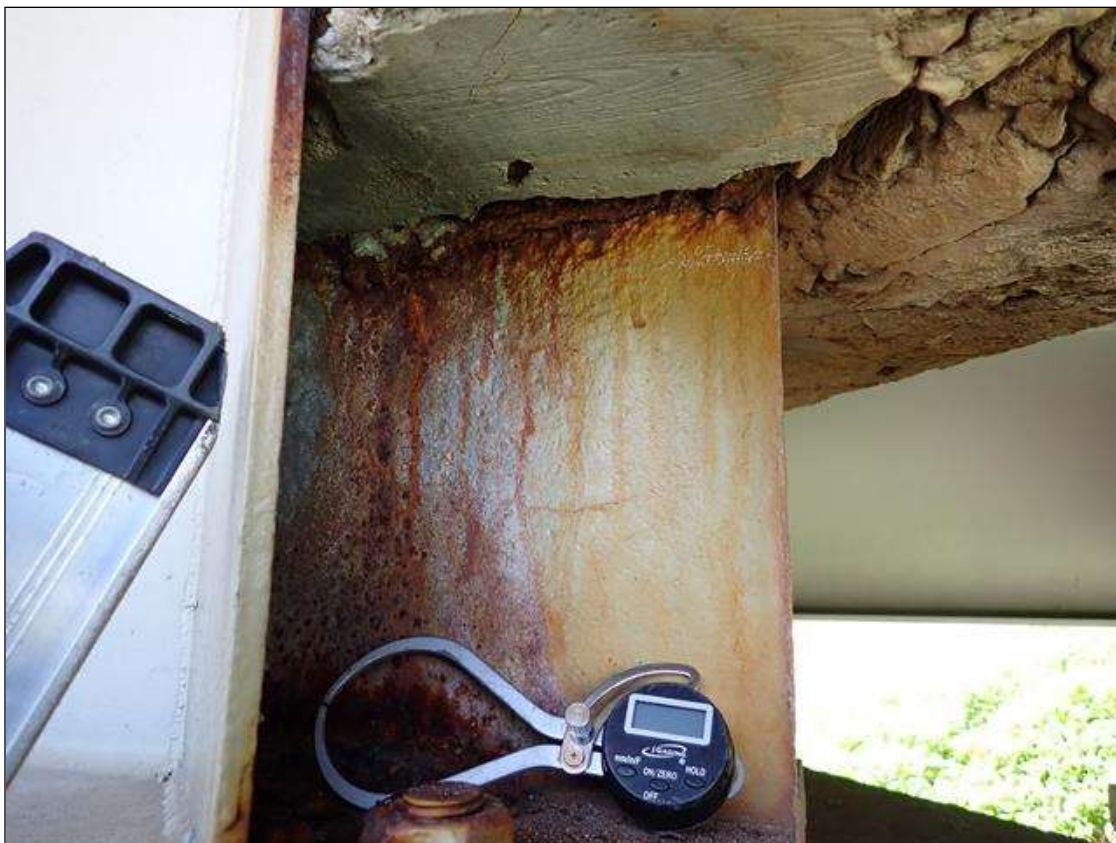
Span 3 Beam 4: at bent 3, web adjacent to end diaphragm, corrosion with section loss (9/16 inch average remaining x 10 inch x 1 inch)
