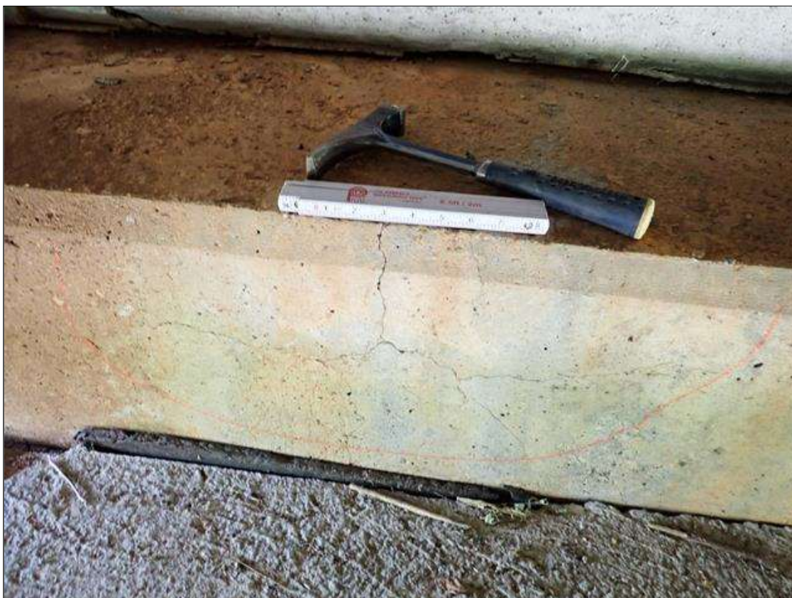
End Bent 2 Cap 1: in bay 1, map cracks (2 foot x 1 foot x up to 1/32 inch)
