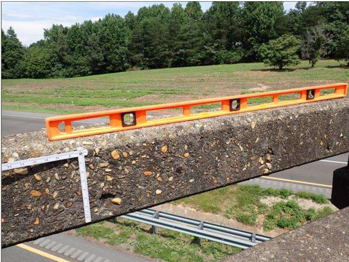
Span 2 Left Bridge Rail: at midspan, (2) spalls (3 inch diameter x 1/2 inch deep) with exposed rusted rebar
