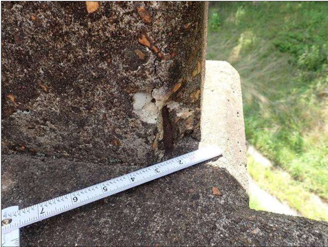
Span 2 Right Bridge Rail: (2) UP TO 4 INCH DIAMETER X 1/2 INCH SPALLS WITH EXPOSED REINFORCING 22 FEET FROM BENT 1 NO SECTION LOSS
