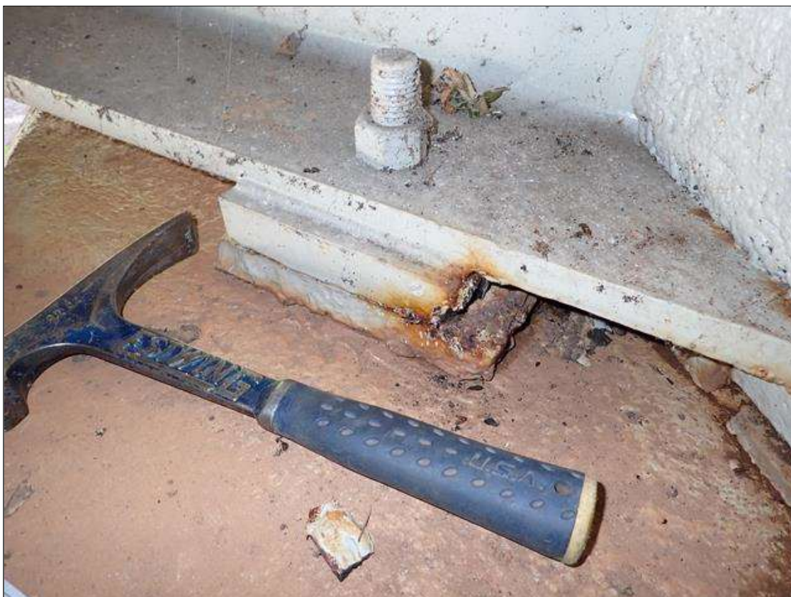
Span 4 Far Bearing 1: corrosion with section loss (up to 1/8 inch loss)
