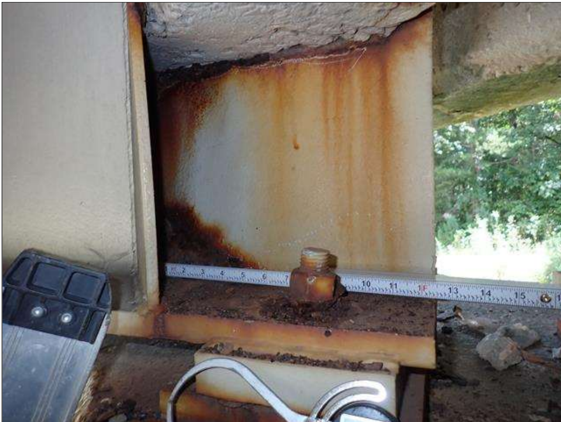
Span 2 Beam 4: at bent 1, corrosion with section loss: web (less than 1/16 inch loss x 1 foot x 10 inch); bottom flange (less than 1/16 inch loss x 1 foot)
