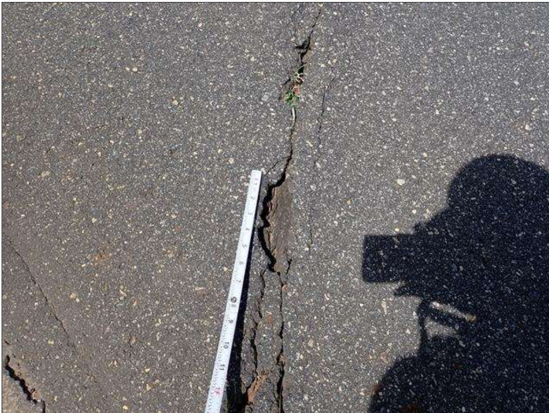
Span 2 Wearing Surface: 35 FEET X UP TO 1/8 INCHES TRANSVERSE CRACK OVER BENT 1 WITH EDGE SPALLS UP TO 3 INCH X 1 INCH DEEP
