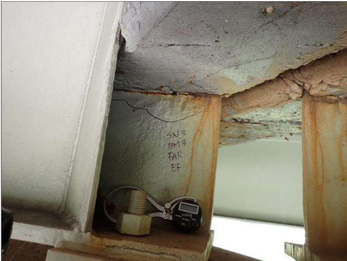
Span 3 Beam 3: (PAR) at bent 3, web adjacent to end diaphragm, corrosion with section loss (7/16 inch average remaining x 10 inch x 2.5 inch)
