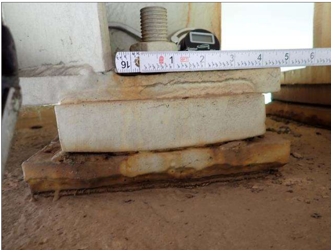
Span 3 Beam 3 - Far Bearing 3: corrosion with section loss (up to 1/8 inch loss)
