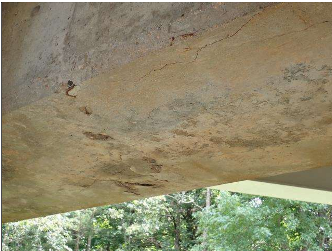
Bent 1 Cap 1: underside between columns 2 and 3, delamination (3 foot x 2 foot) with cracks (up to 1/16 inch)
