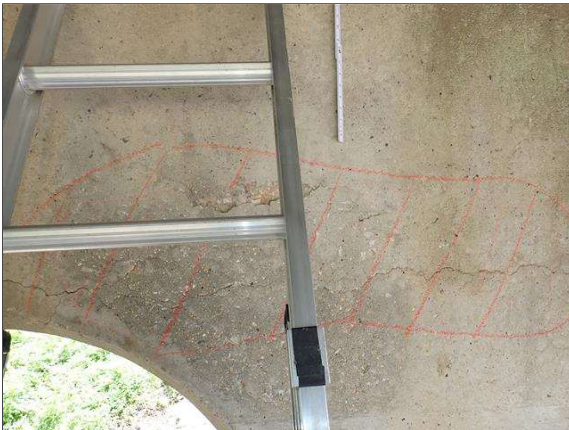
Bent 1 Cap 1: NORTH FACE OF CAP HAS A DELAMINATED/SPALLED AREA ALONG THE BOTTOM EDGE AT COLUMN 2 4 FOOT X 1.5 FOOT X 1/2 INCH DEEP WITH CRACKS UP TO 1/32 INCH
