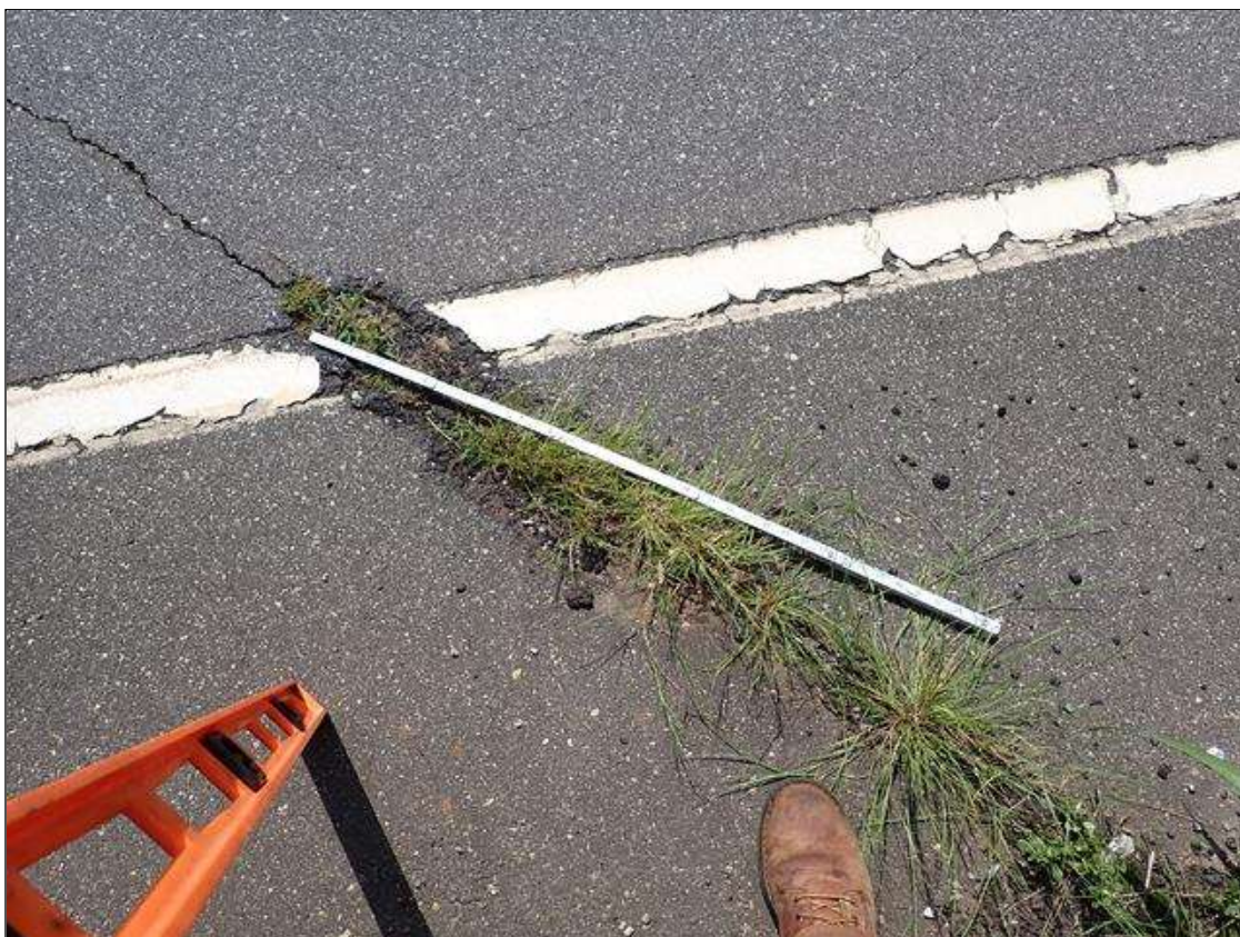
Span 3 Wearing Surface: 35 FEET X UP TO 1/8 INCHES TRANSVERSE CRACK WITH EDGE SPALLS UP TO 2 FOOT X 4 INCH X 1 INCH DEEP WITH VEGETATION GROWTH OVER BENT 2
