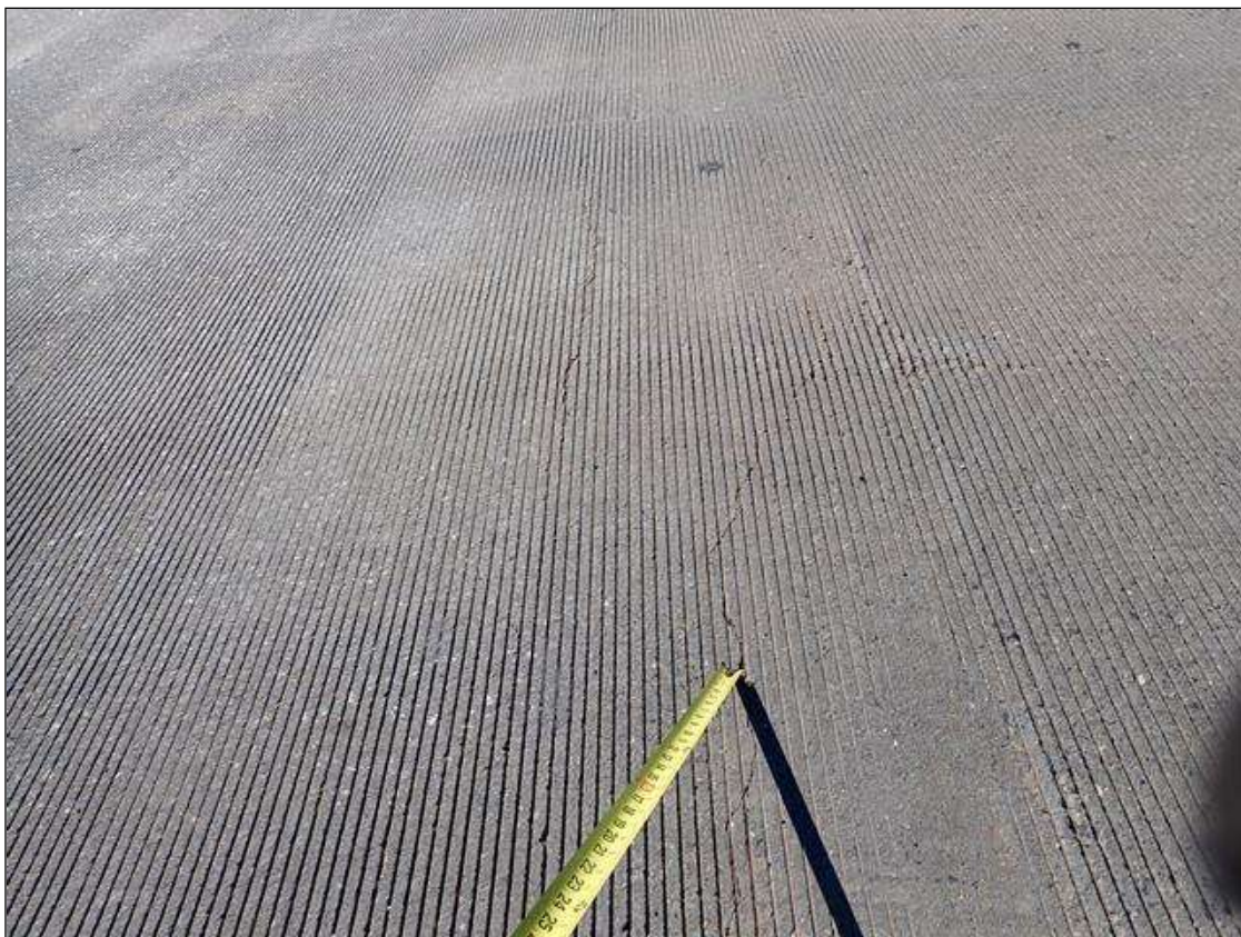
Span 2 Deck: multiple full width transverse cracks up to 1/16 inch wide, near bent 1, in south bound lanes.
