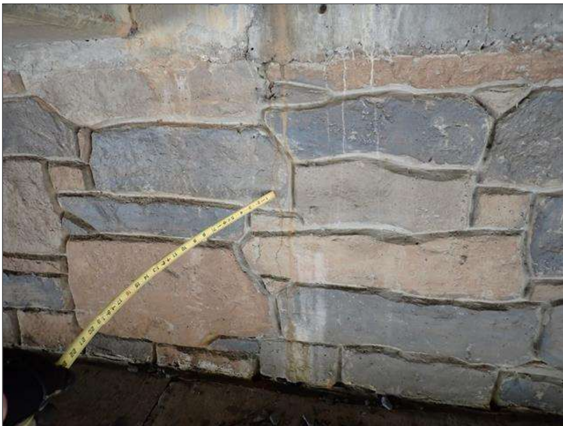
End Bent 1 Cap 1: below bay 6, vertical crack (1/64 inch x full height)
