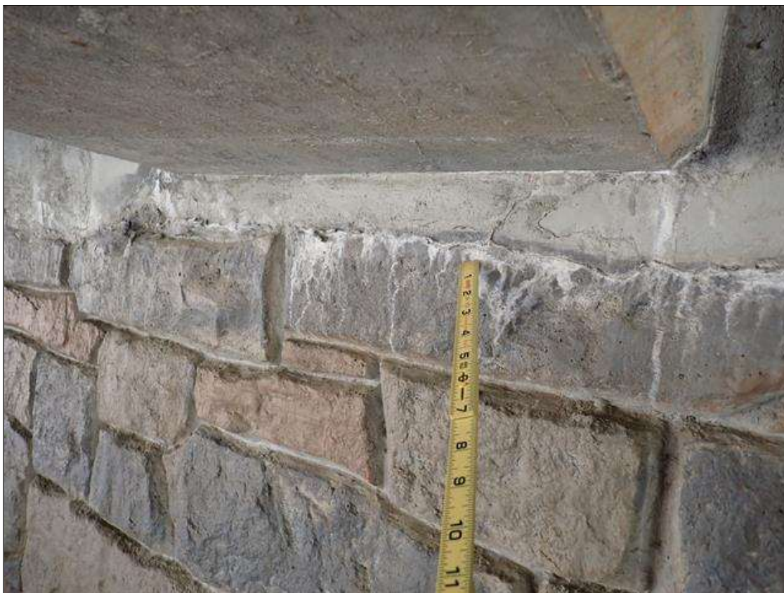
End Bent 1 Cap 1: below beam 8, at construction joint with abutment, efflorescence (2 feet)
