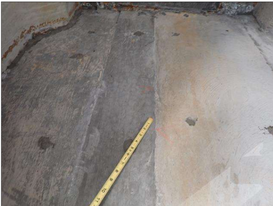
End Bent 2 Abutment: at bay 6, at construction joint, vertical crack, full height x up to 0.012 inch
