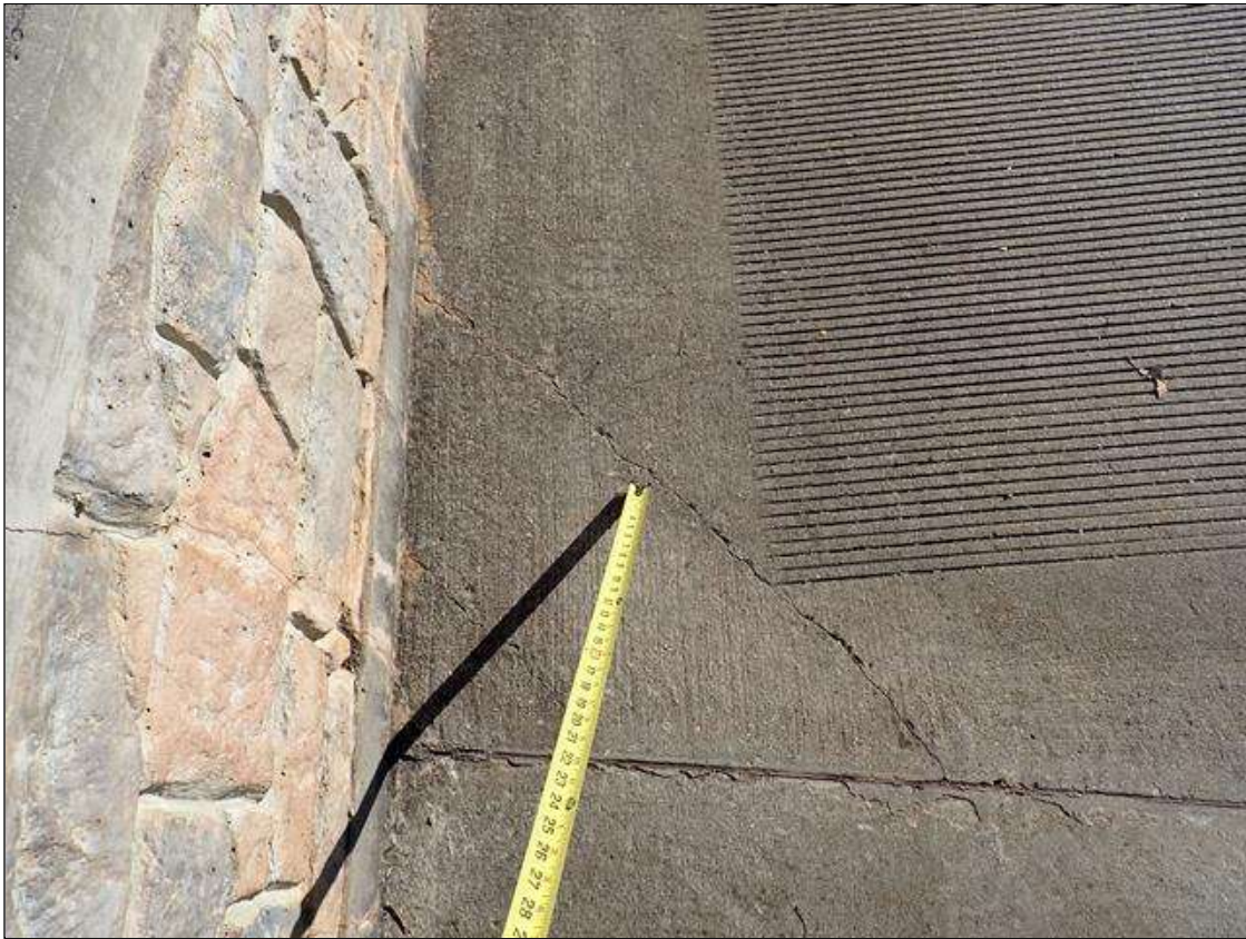
Approach 1 : 2 diagonal x 1/16 inch cracks in far right corner of approach slab, 40 inches long and 16 inches long
