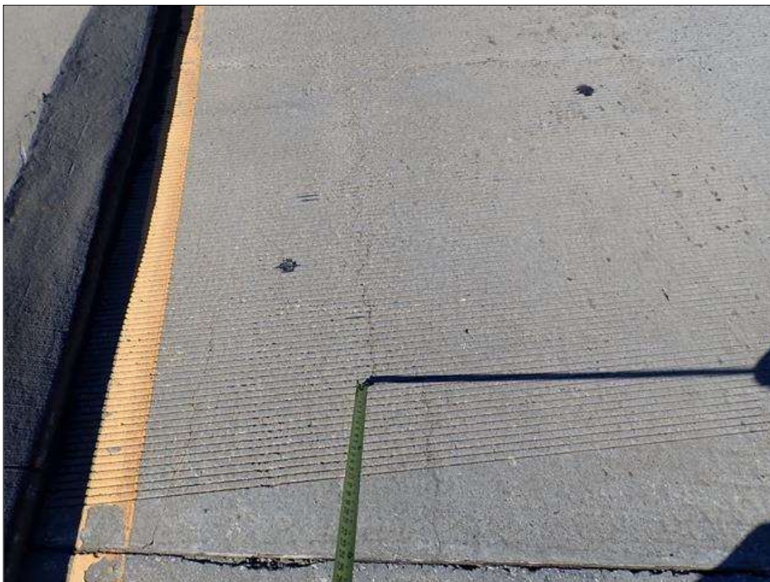
Span 1 Deck: 3 - longitudinal cracks up to 1/32 inch wide x up to 4 feet long, extending from end bent 1 joint, in northbound lanes.
