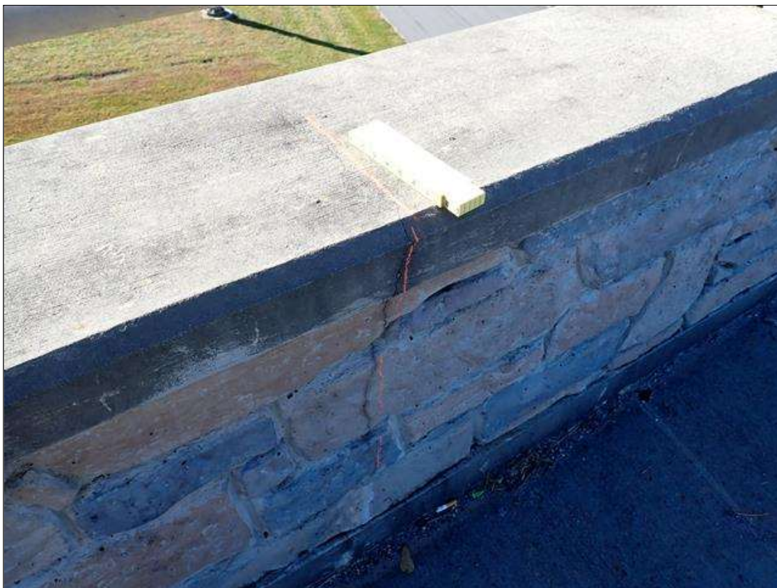
Span 1 Left Bridge Rail: up to full height x 1/64 inch vertical cracks in top of rail extending down face
