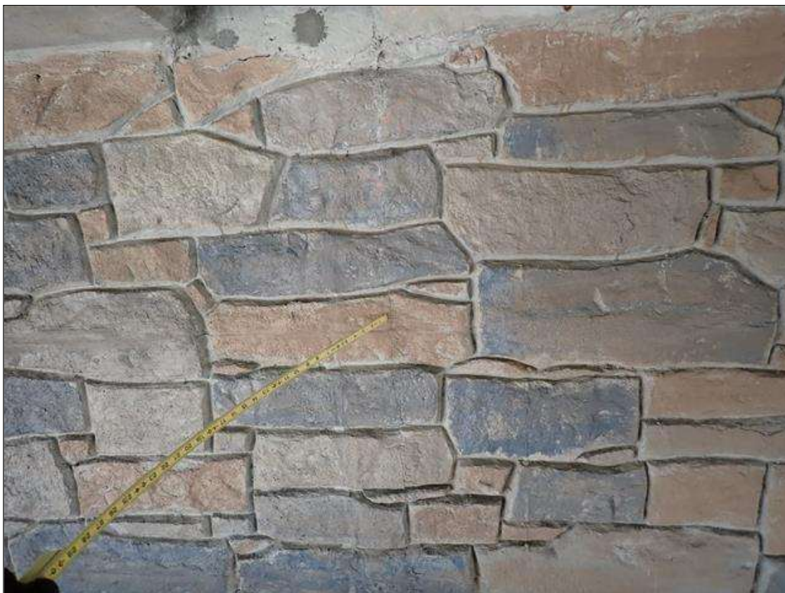
End Bent 2 Cap 1: vertical crack up to 1/32 inch wide, in front face, below bay 6.
