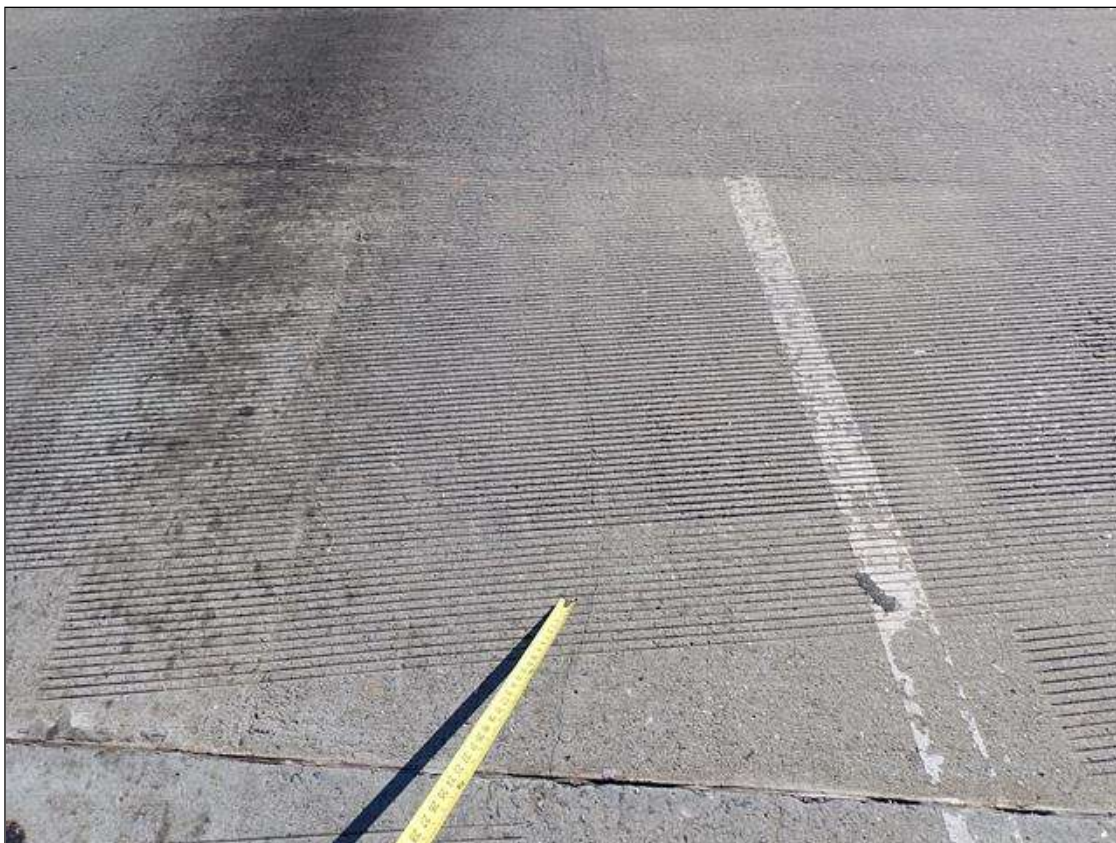
Span 2 Deck: 3 - longitudinal cracks up to 1/32 inch wide x up to 4 feet long, in south bound lanes, at end bent 2.
