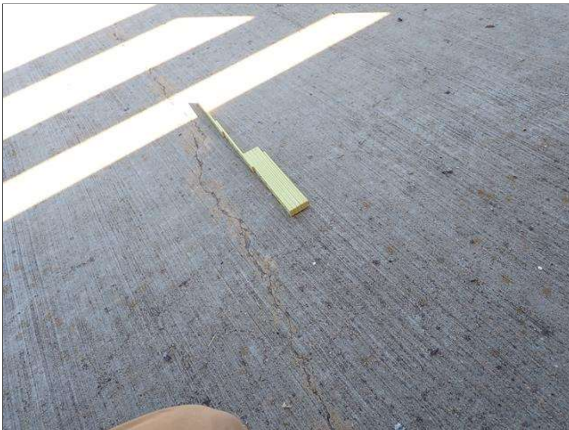
Span 2 Left Bridge Rail: sidewalk at random, transverse cracks (up to 1/16 inch x 9 feet)
