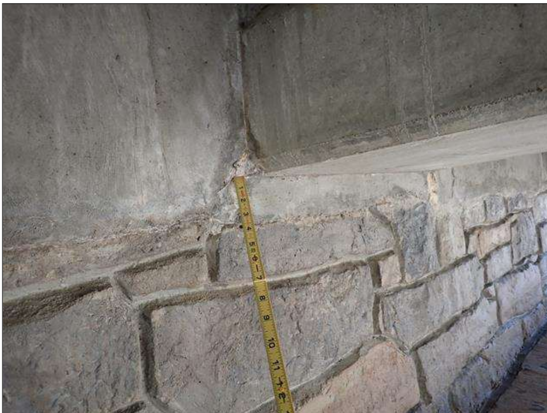
End Bent 1 Abutment: at multiple beams, at bottom flange, diagonal crack (hairline x 4 inch) with efflorescence
