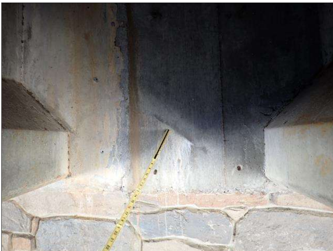
End Bent 1 Abutment: bay 6 closure pour, diagonal crack (hairline x 1 foot) with efflorescence
