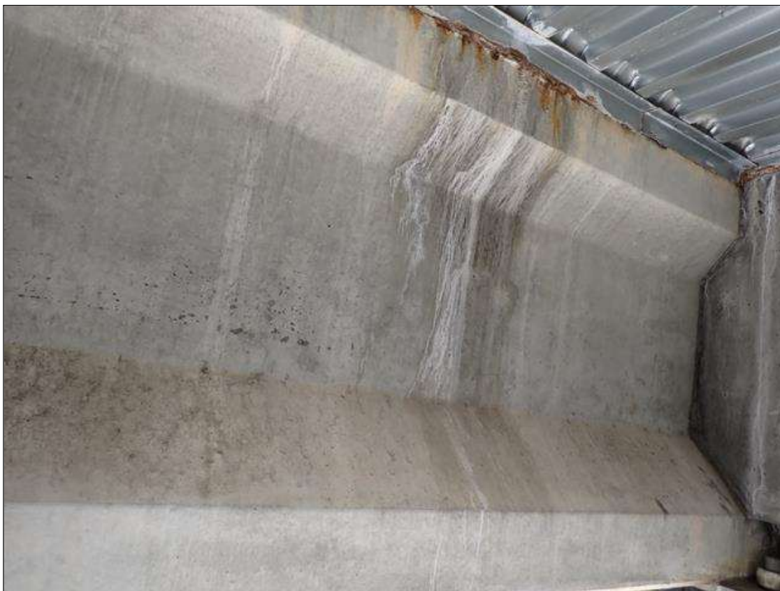
Span 1 Beam 1: near bent 1, top flange, right face, efflorescence (2 feet)
