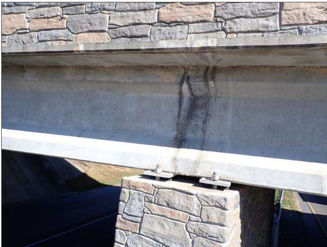
Span 1 Beam 1: bent 1 closure pour, at seams, efflorescence
