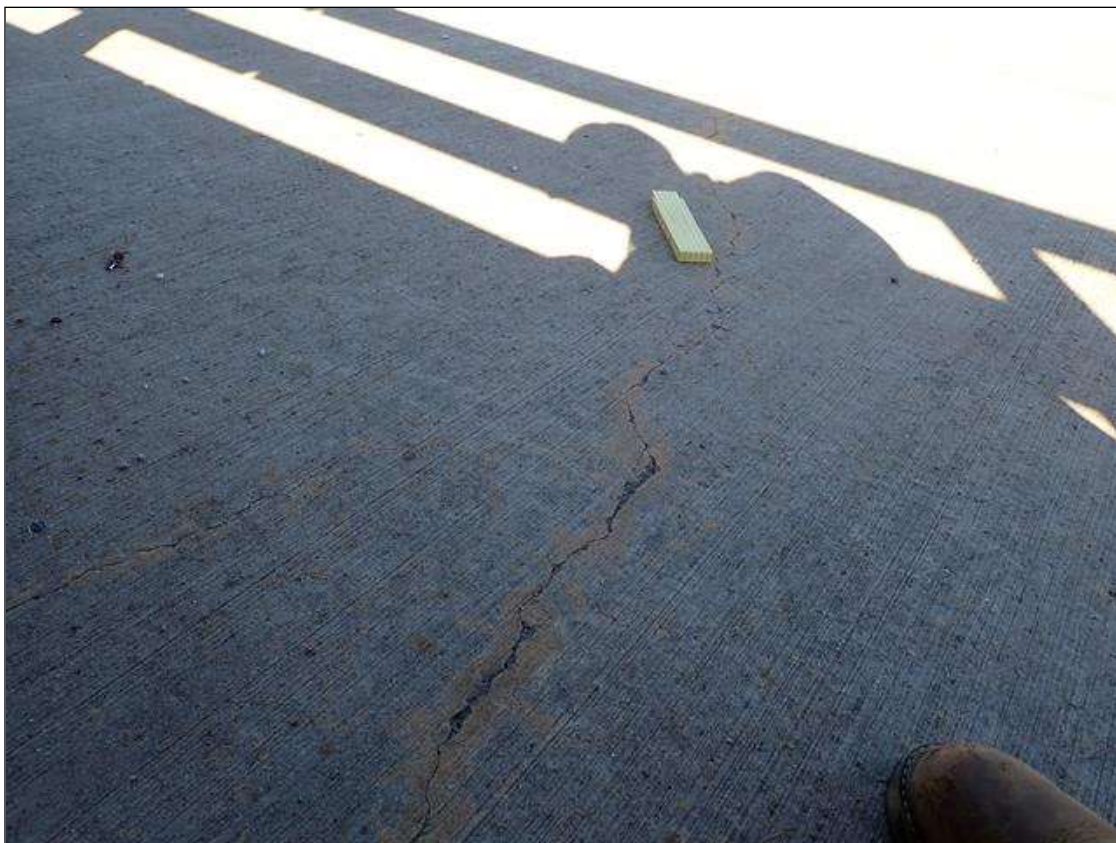
Span 1 Left Bridge Rail: sidewalk at random, transverse cracks (up to 1/16 inch x 9 feet)
