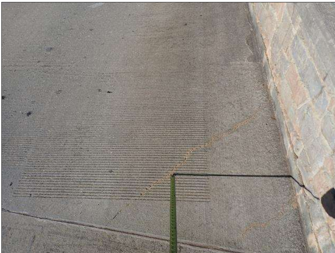
Approach 2 : 2 diagonal x 1/16 inch cracks in near right corner of approach slab, 58 inches long and 20 inches long
