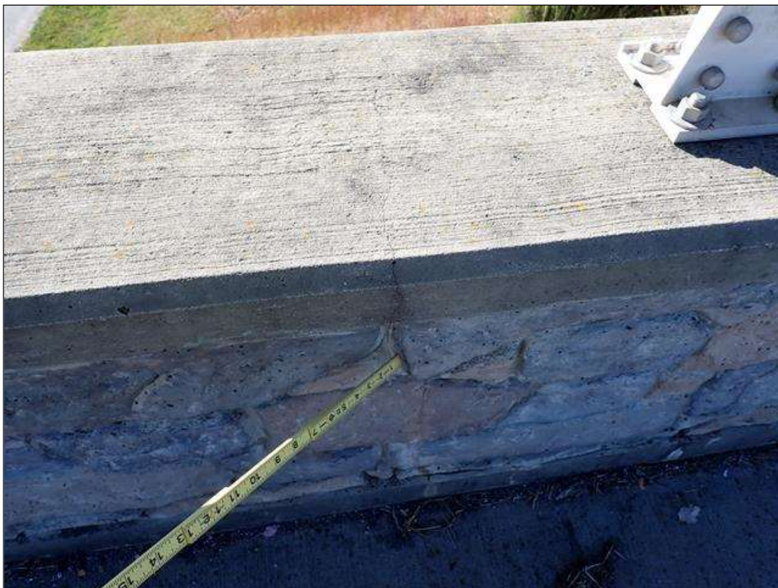
Span 2 Left Bridge Rail: up to full height x 1/64 inch in top of rail extending down face
