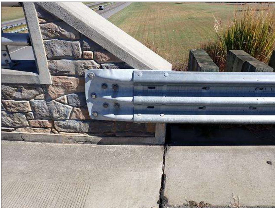
southeast guardrail attachment
