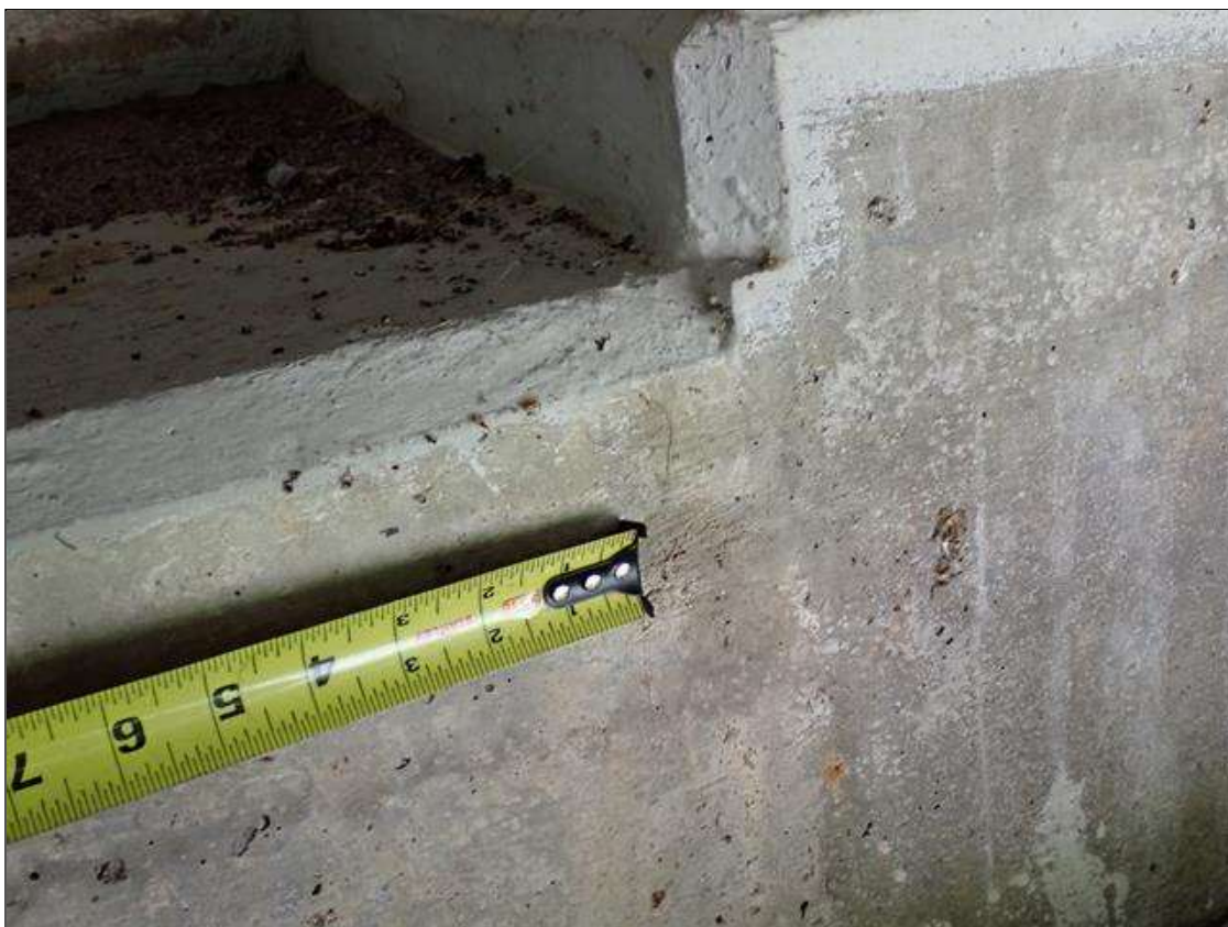
End Bent 1 Cap 1: along length, multiple vertical cracks, up to 8 inch x hairline
