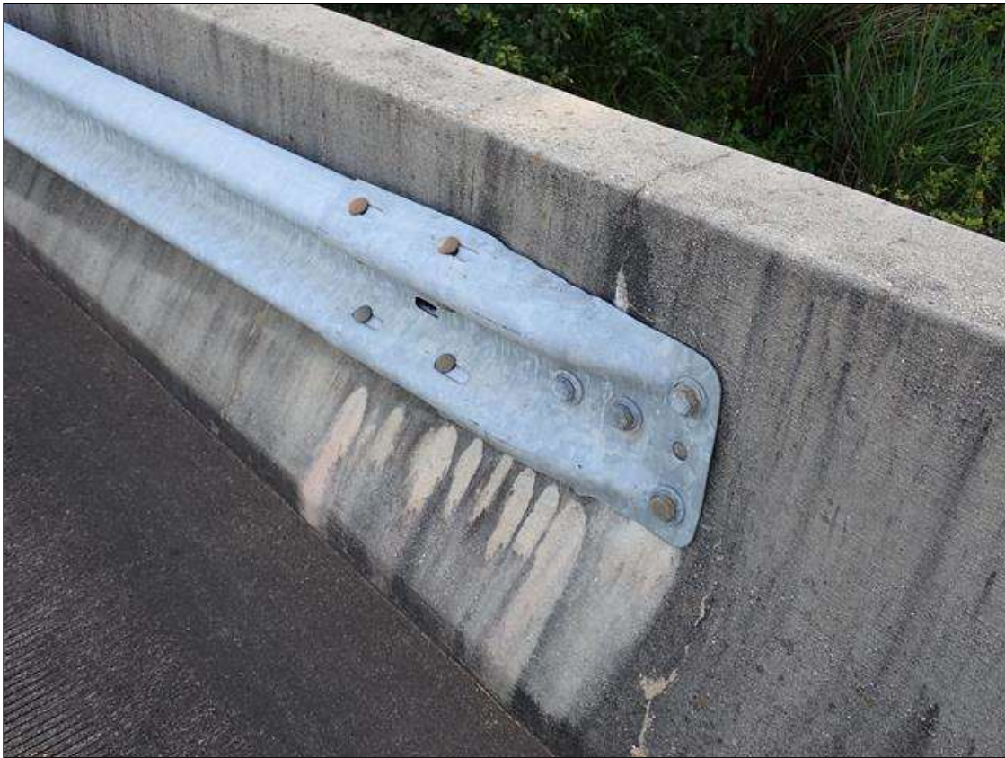
northeast guardrail attachment
