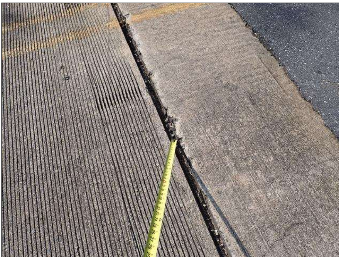
Approach 1 : along end bent 1 joint, edge spalls (up to 4 inch x 2 inch x 1 inch deep)
