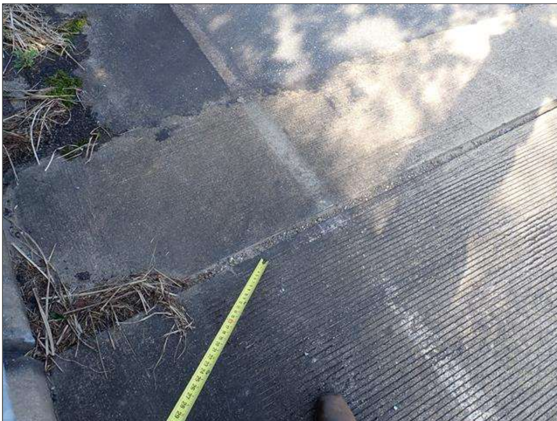
Span 1 End Bent 1 Joint: LOOSE GRAVEL DEBRIS AT RANDOM THROUGHOUT
