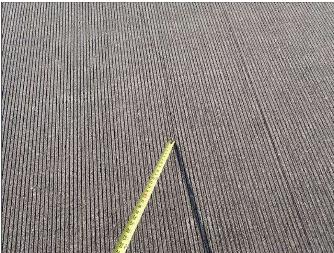
Span 1 Deck: southbound lane, near bent 1, transverse crack (1/32 inch x 6 feet)
