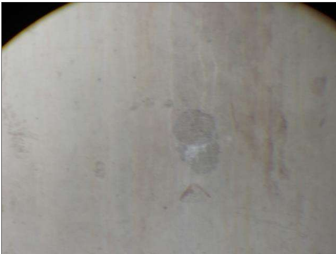
Bent 1 Pile 2: north face, near cap, efflorescence
