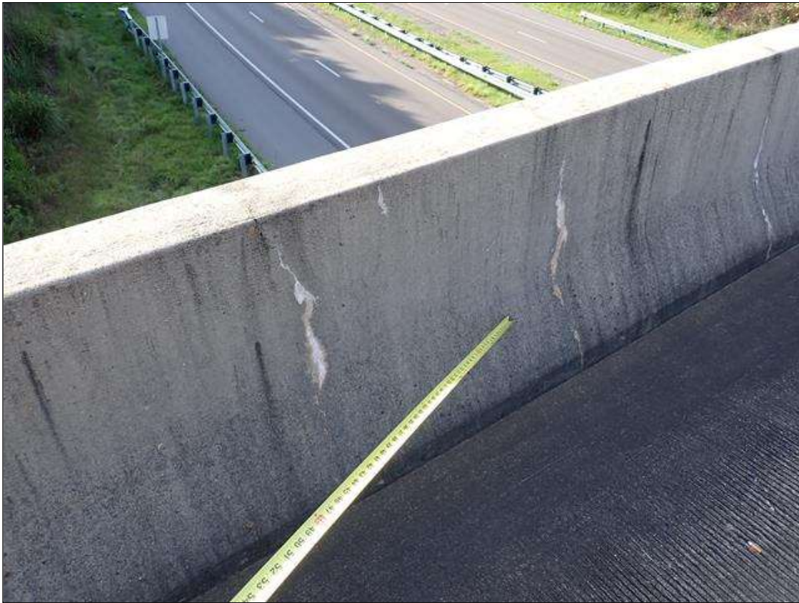
Span 2 Right Bridge Rail: 27 - VERTICAL, HORIZONTAL AND WRAP AROUND CRACKS UP TO 1/32 INCH WITH EFFLORESCENCE AT RANDOM THROUGHOUT
