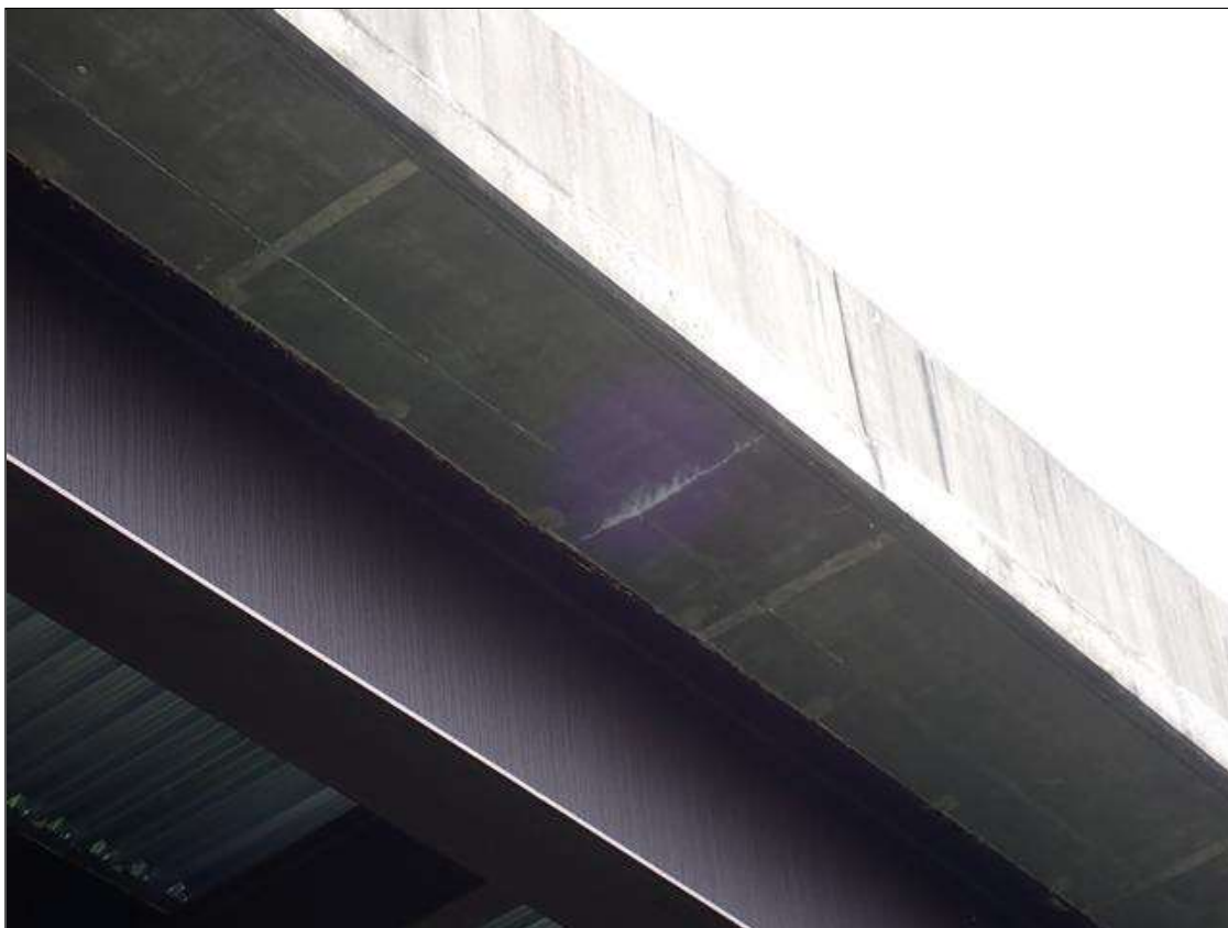
Span 1 Deck: TRANSVERSE CRACKS UP TO 1/64 INCH WITH EFFLORESCENCE UNDERSIDE OF WEST OVERHANG AT RANDOM THROUGHOUT.
