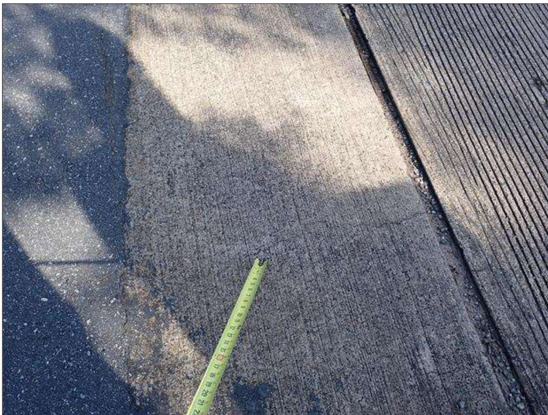
Approach 1 : throughout approach slab, longitudinal cracks (up to 1/32 inch x 2.5 feet) and areas of map cracks (hairline) at random
