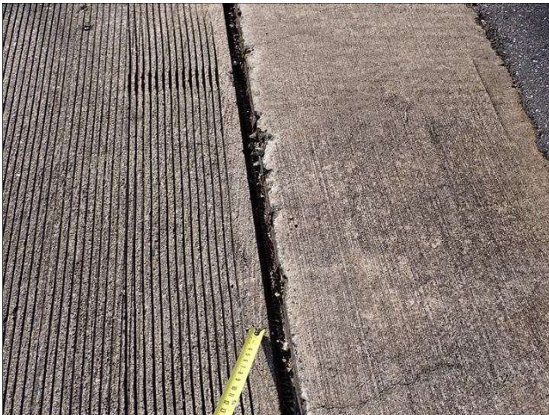
Span 1 End Bent 1 Joint: (not found 2023) along length of joint at random throughout, adhesion loss greater than 50 percent
