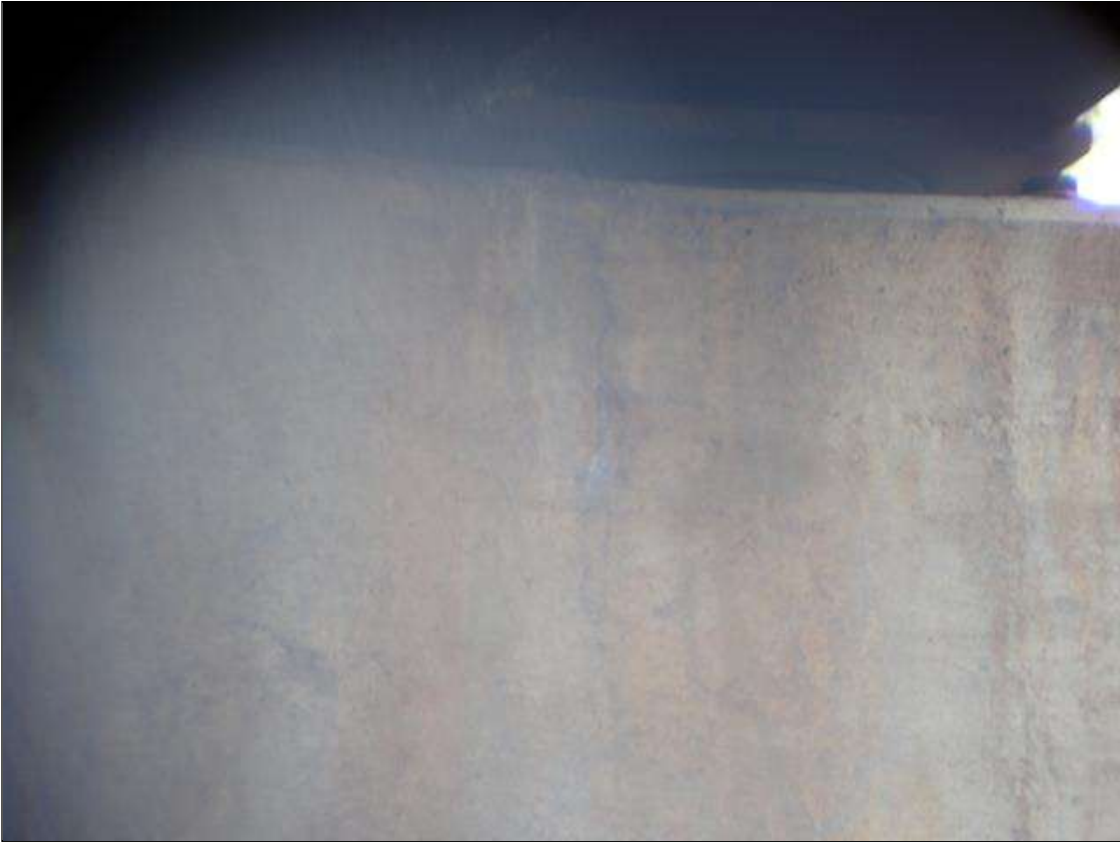
Bent 1 Cap 1: SCATTERED VERTICAL AND DIAGONAL CRACKS UP TO 1/32 INCH, SOME WITH EFFLORESCENCE, AT RANDOM THROUGHOUT ALL FACES.
