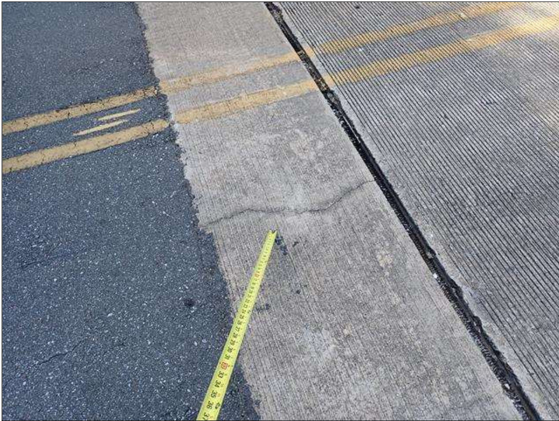
Approach 2 : throughout approach slab, longitudinal cracks (up to 1/32 inch x 2.5 feet) and areas of map cracks (hairline) at random
