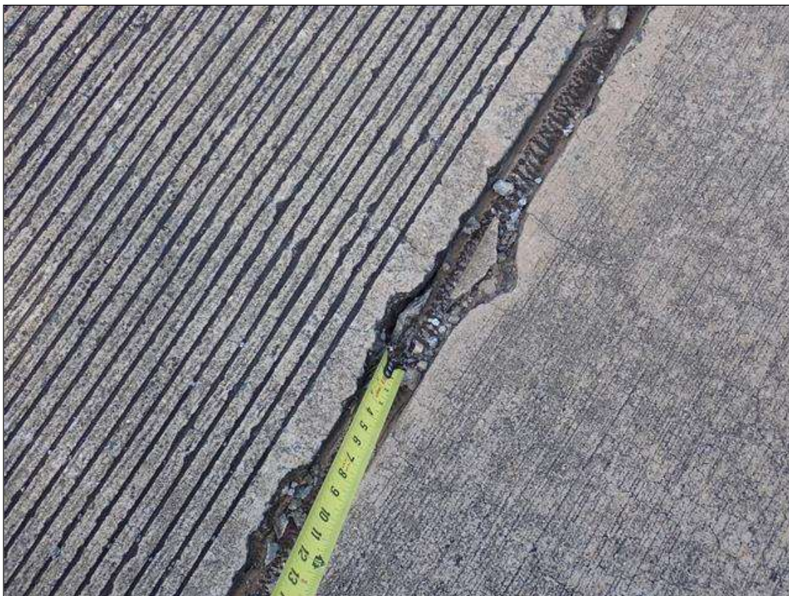
Span 2 End Bent 2 Joint: along length of joint at random throughout, adhesion loss greater than 50 percent
