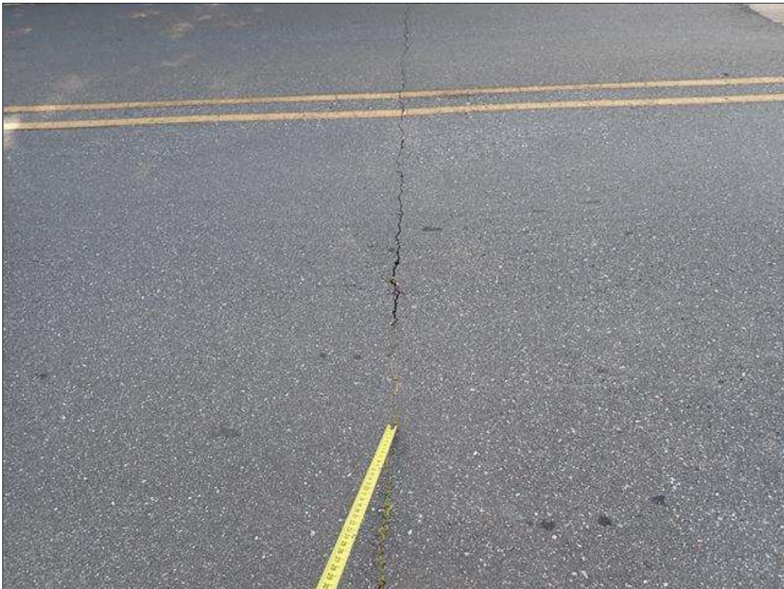
south and north approach asphalt, adjacent to approach slabs, transverse cracks (up to 1/4 inch x full width of roadway)
