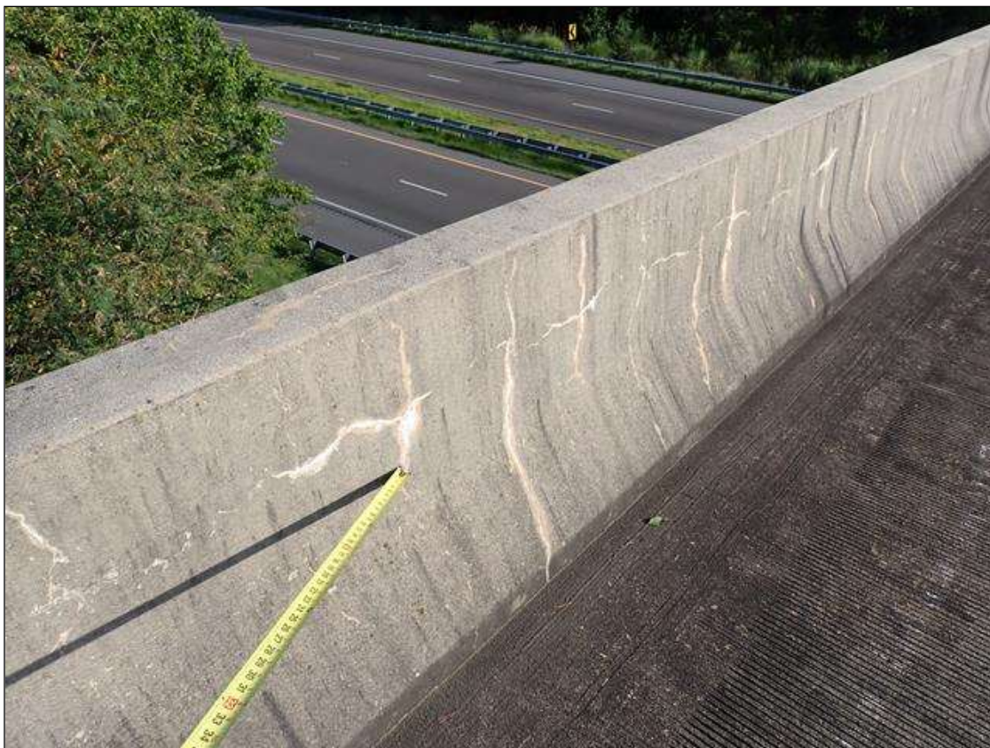
Span 1 Left Bridge Rail: (PAR) VERTICAL, horizontal AND WRAP AROUND CRACKS UP TO 1/32 INCH WITH EFFLORESCENCE AND EFFLORESCENCE BUILDUP AT RANDOM THROUGHOUT
