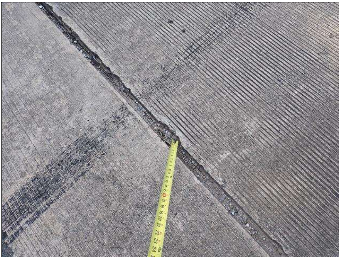
Span 2 End Bent 2 Joint: along the length of the joint, edge spalls (up to 8 inch x 1 inch x 1 inch deep)
