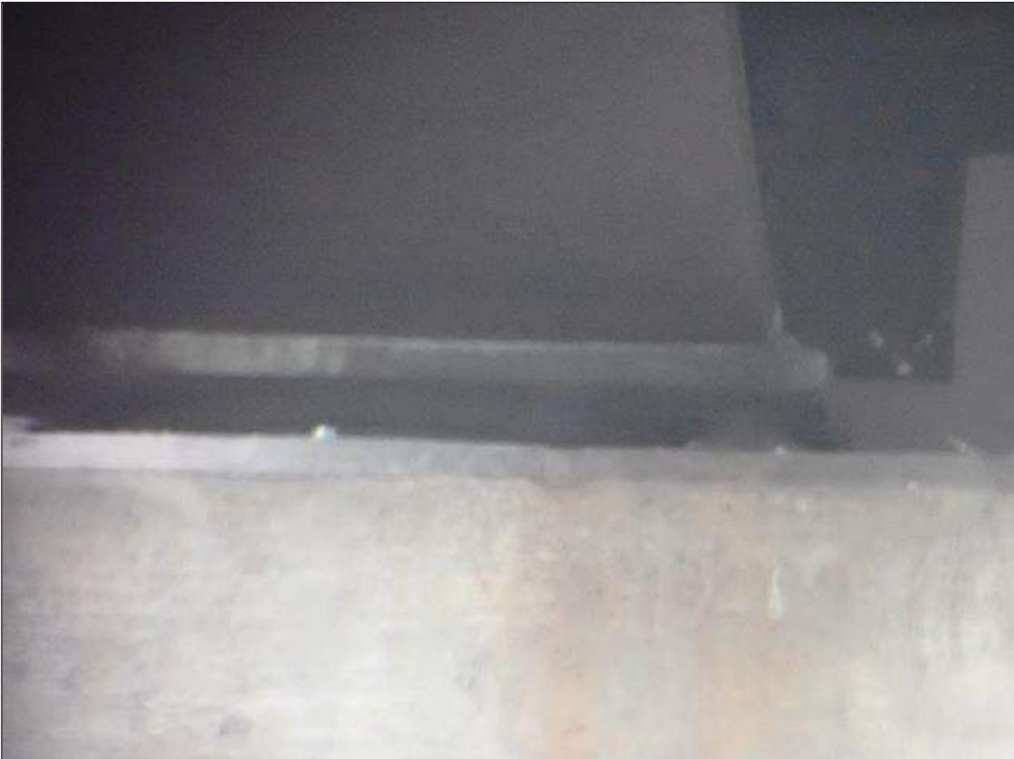
Span 1 Beam 4 - Intermediate Bearing 4: FRECKLED RUST
