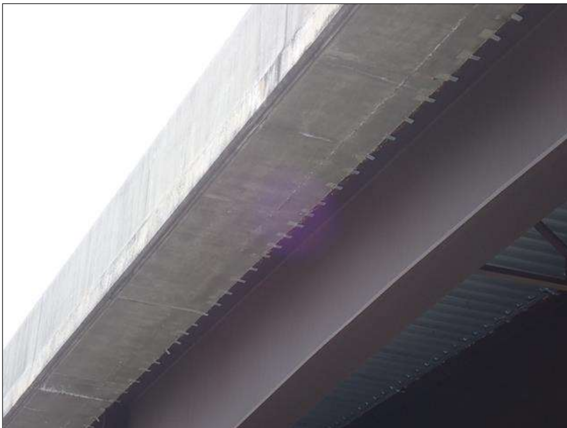
Span 2 Deck: TRANSVERSE CRACKS UP TO 1/64 INCH WITH EFFLORESCENCE UNDERSIDE OF EAST OVERHANG AT RANDOM THROUGHOUT.
