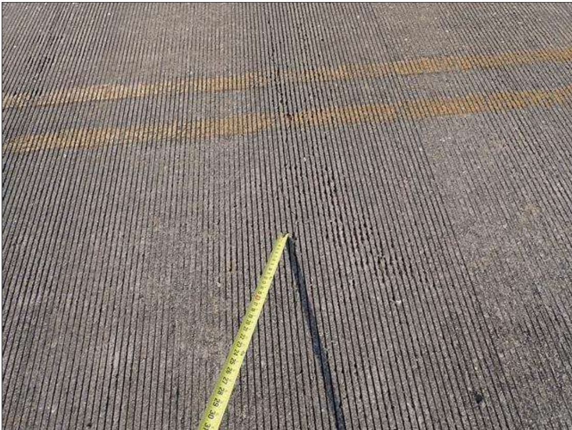
Span 2 Deck: SCATTERED TRANSVERSE CRACKS UP TO 1/32 INCH AT RANDOM THROUGHOUT top of deck
