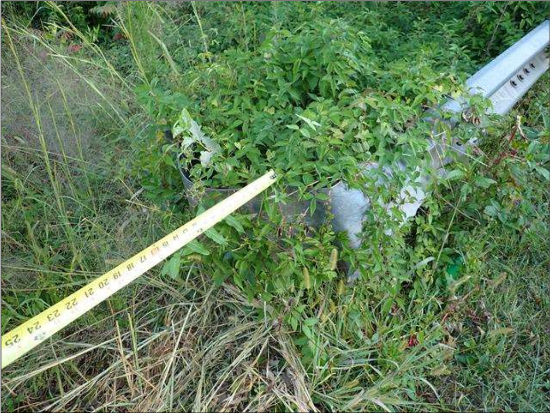
(PAR) southwest guardrail termination, impact damage (1 foot)
