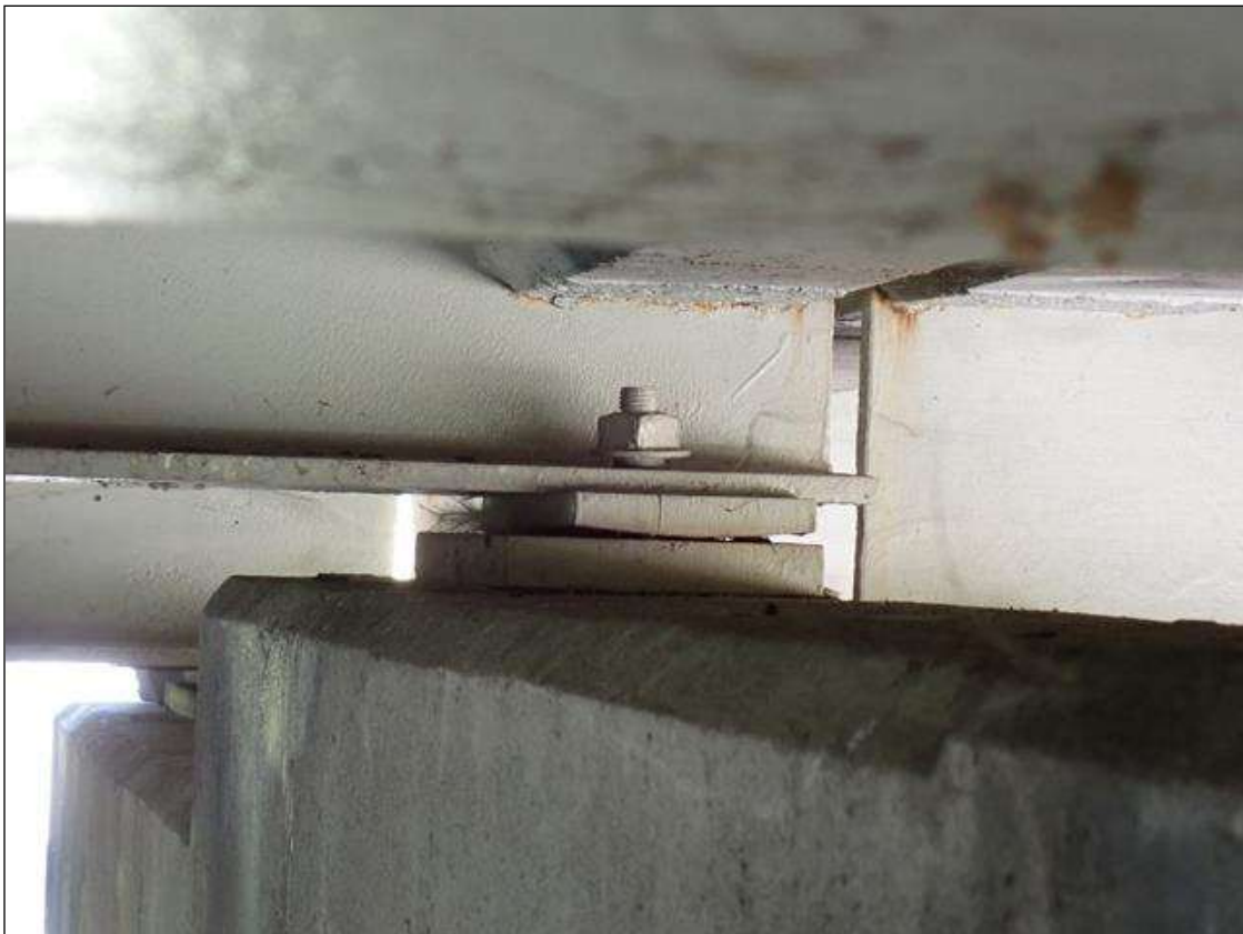
Span 1 Beam 2 - Far Bearing 2: (not found 2023) surface rust.
