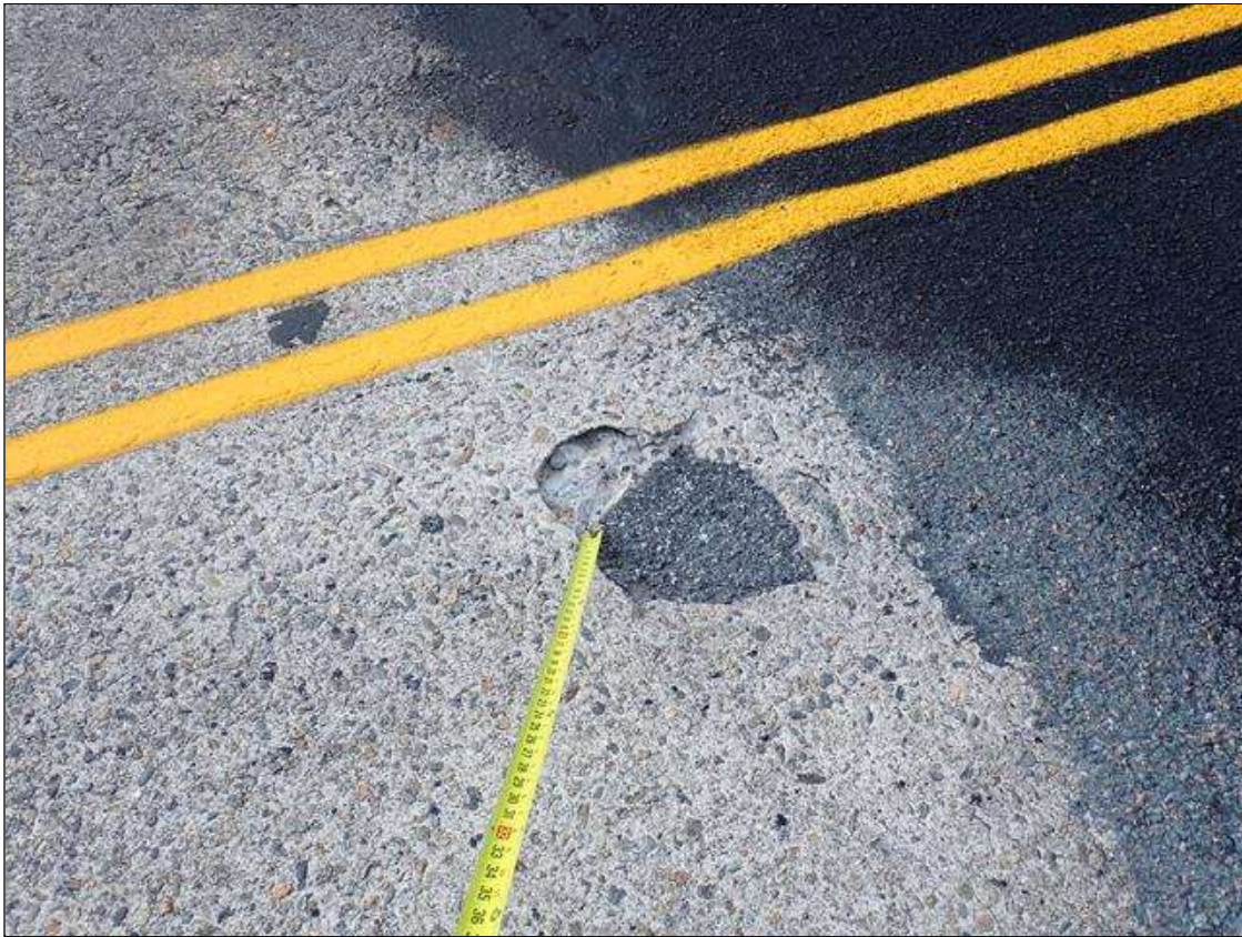
Span 1 Deck: southbound lane, near end bent 1, partially patched spall (18 inch x 15 inch x 1.5 inch deep)
