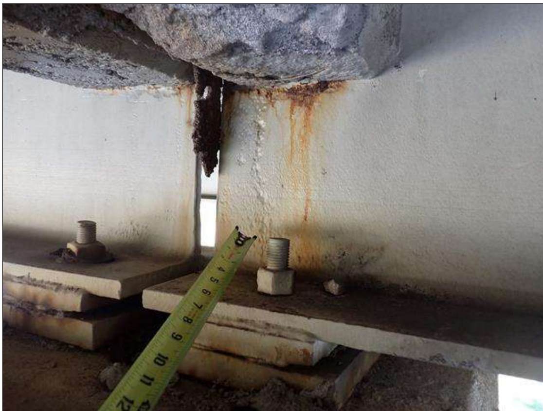
Span 2 Beam 3: at bent 2, web over bearing, painted over pitting (1/8 inch deep x 7 inch x 10 inch) with corrosion reinitiated
