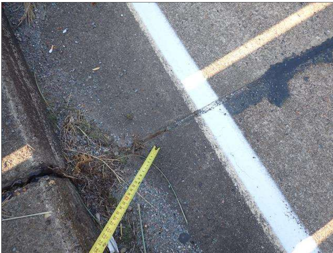
Span 2 Expansion Joint at Bent 1: both shoulders, seal damage (up to 1 inch deep)
