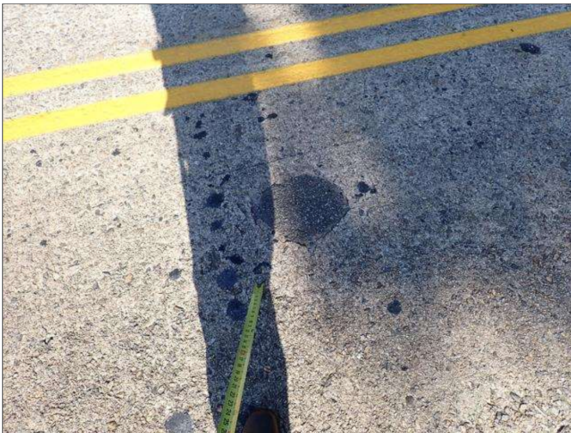
Span 4 Deck: 18 inch diameter sound asphalt patch, in northbound lane, near midspan, with associated adjacent delaminations and broken asphalt
