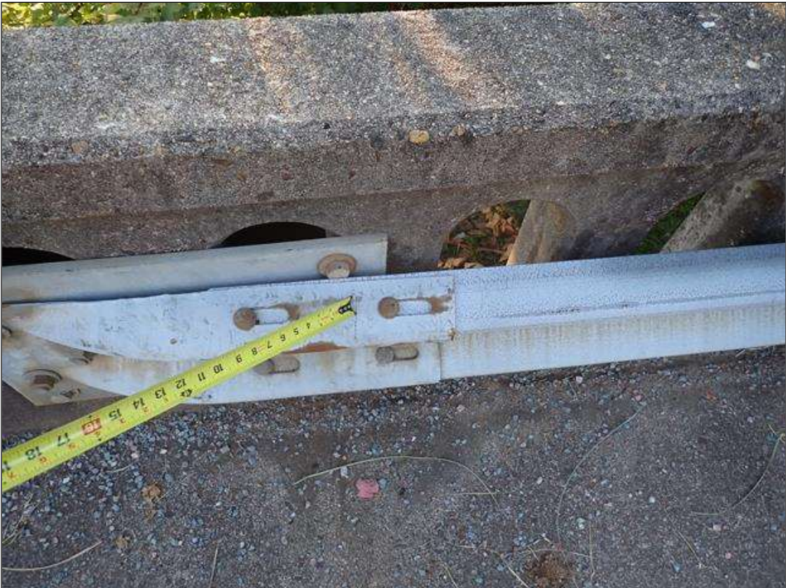
(PAR) southeast guardrail attachment, improper lap
