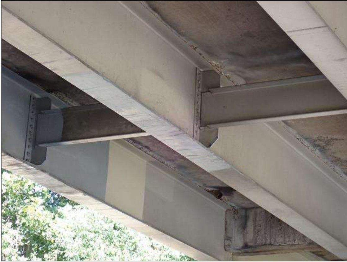
Span 3 Beam 2: (PAR) 2023 area repainted with new impact scrapes/gouges up to 1/8 inch deep; previously noted as: SUPPLEMENTAL INSPECTION IMPACT DAMAGE 2022.: beam 2 span 3 deflected upward 1/2 inch at 19.5 inches from bent 2 for a length of 4 feet, with scrapes on bottom flange
