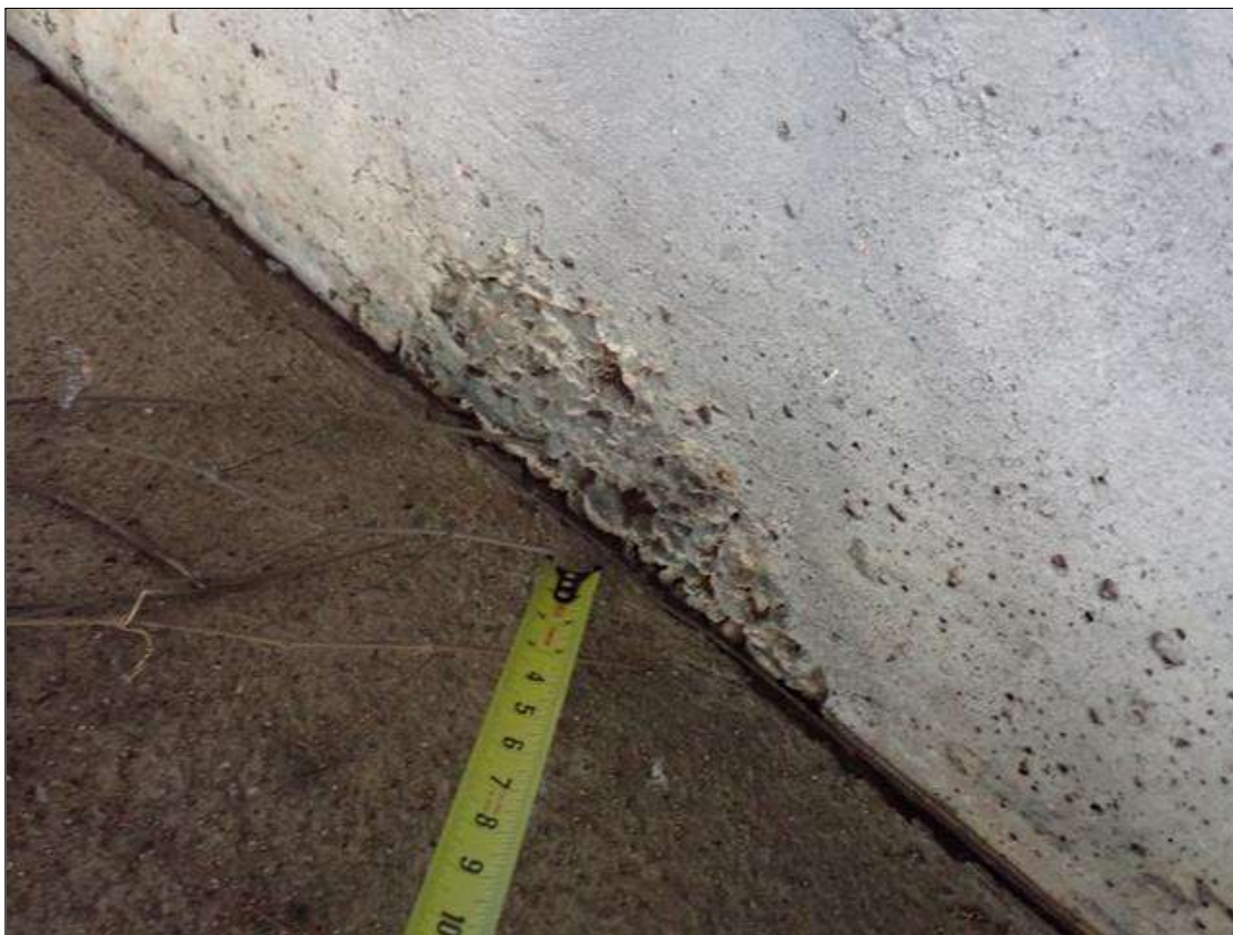
End Bent 1 Cap 1: 14 inch x 6 inch x 1 inch deep area of honeycombing in face of cap under beam 2
