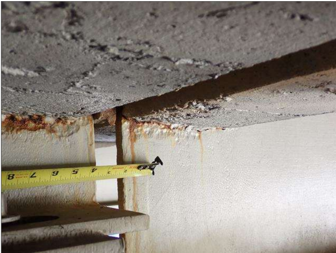
Span 2 Beam 3: (PAR) at bent 1, web adjacent to diaphragm, painted over section loss (3/8 inch average remaining x 6 inch x 1 inch) with corrosion reinitiated
