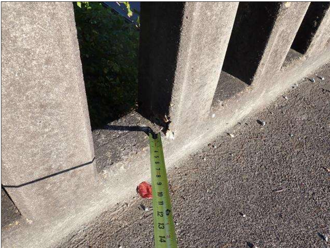
Span 1 Left Bridge Rail: 5 - spalls with exposed reinforcing up to 3 inch x 1 inch x 1/2 inch deep, in traffic and outside faces, at random., no section loss noted.
