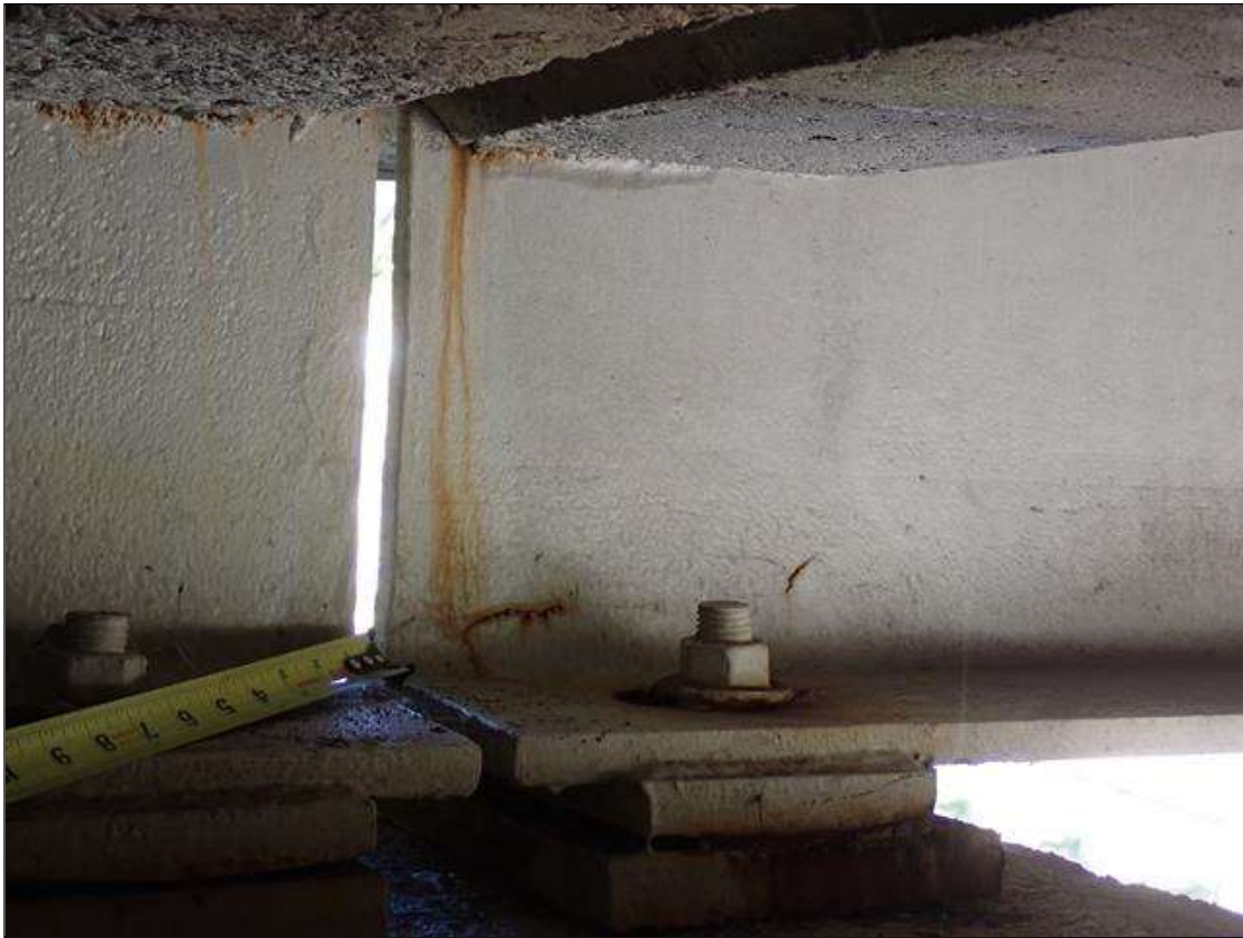
Span 2 Beam 1: (PAR) at bent 1, web adjacent to diaphragm, painted over section loss (3/8 inch average remaining x 7 inch x 1 inch); painted over pitting: lower web, painted over pitting (up to 1/16 inch deep x 1 foot x 6 inch) with corrosion reinitiated
