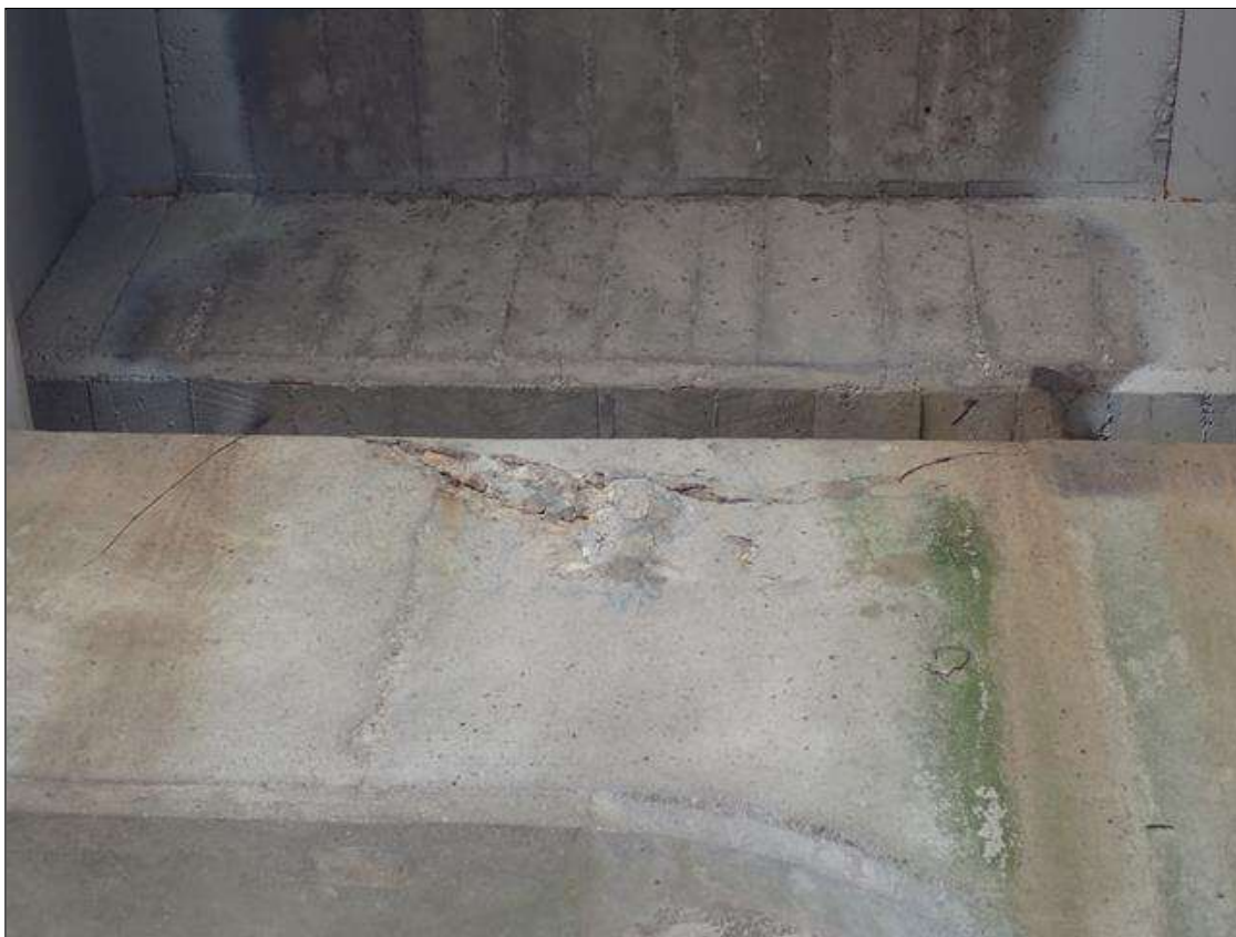
Bent 1 Cap 1: in north face under bay 3, delamination/spall [up to 3 feet x up to 15 inch x 1.5 inch deep]
