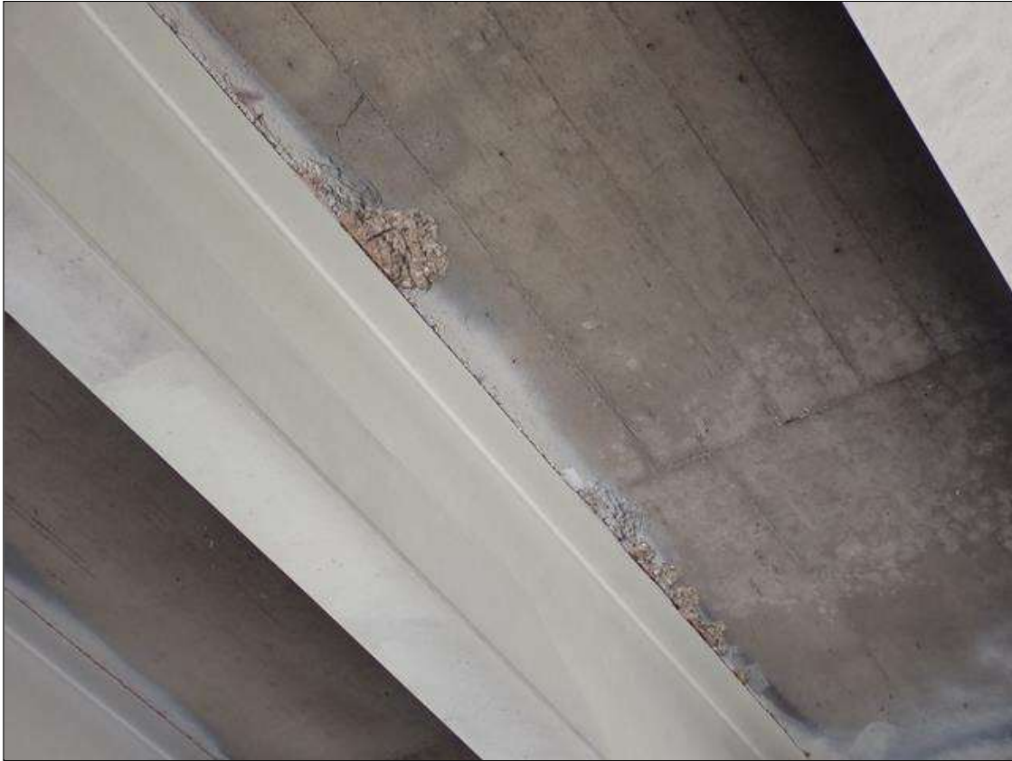
Span 3 Deck: (PAR) up to 4 feet long x 10 inch wide x 1 inch deep spalling, some with exposed rusted rebar, in underside of deck, along edges of beam 3.
