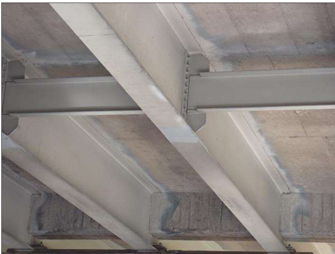
Span 3 Beam 4: 2023 area repainted; previously noted as: SUPPLEMENTAL INSPECTION IMPACT DAMAGE 2022.: Beam 4 Span 3 has scrapes to bottom flange at 16.75 feet from bent 3 for a total length of 1 foot
