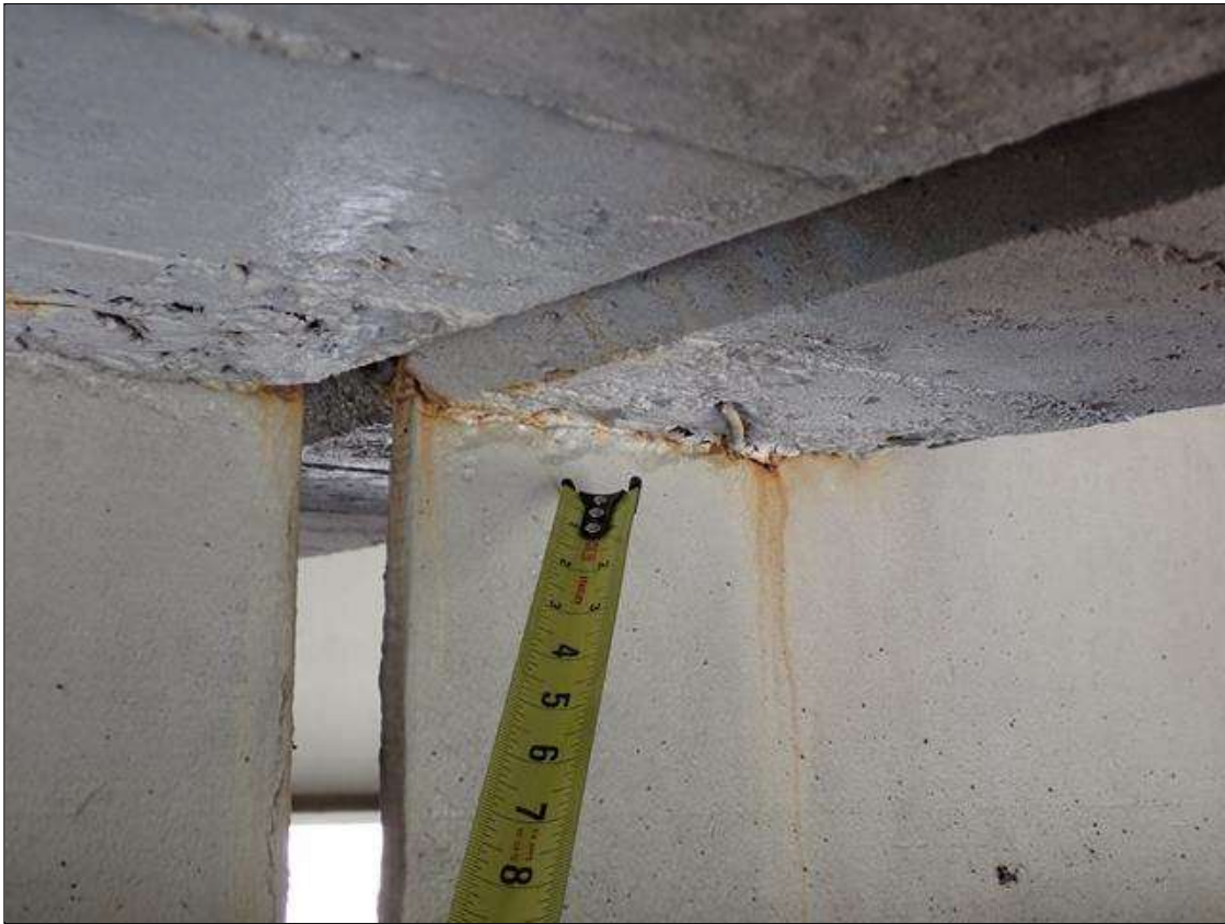
Span 3 Beam 4: (PAR) at bent 2, web adjacent to diaphragm, painted over section loss (3/8 inch average remaining x 6 inch x 1 inch) with corrosion reinitiated
