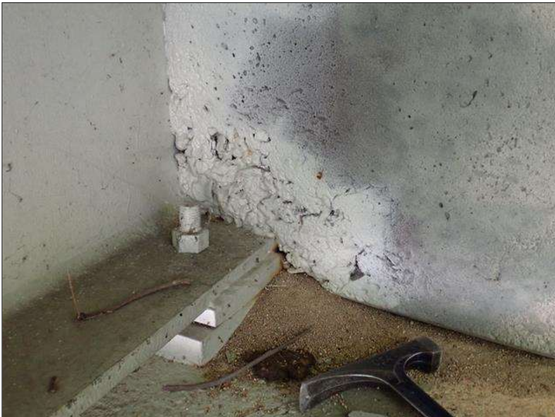
End Bent 1 Abutment: left overhang, adjacent to beam 1, poor consolidation (12 inch x 8 inch x 1 inch deep)
