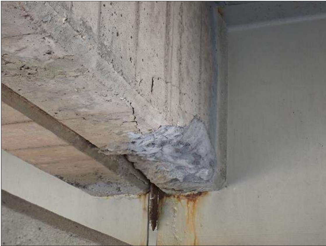
Span 2 Beam 2: 2 foot x full width x 6 inch deep spall/delamination in end diaphragm at bent 2, under bay 2 adjacent to beam 3.
