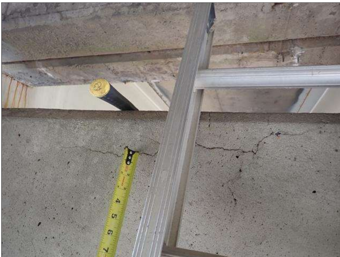
Bent 2 Cap 1: south face, below bays 1-3, longitudinal cracks (up to 1/32 inch x 5 feet) with adjacent map cracks (hairline)
