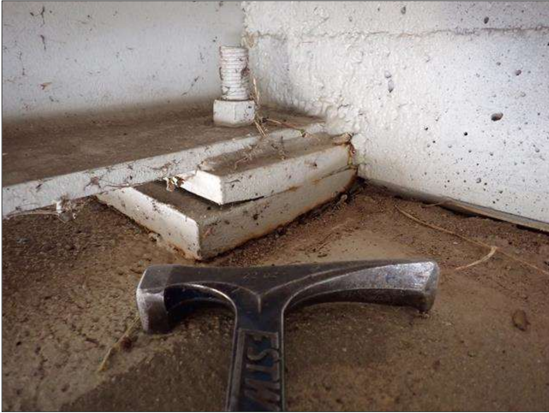
Span 4 Beam 4 - Far Bearing 4: freckled rust
