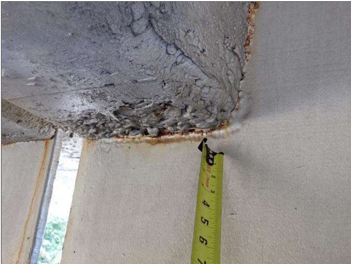
Span 2 Beam 5: (PAR) at bent 2, web adjacent to diaphragm, painted over section loss (3/8 inch average remaining x 9 inch x 1 inch); east top flange, painted over pitting (up to 1/8 inch deep x 6 inches x 4 inches) with corrosion reinitiated
