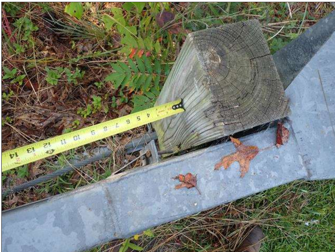
(PAR) southeast guardrail termination, disconnected termination block
