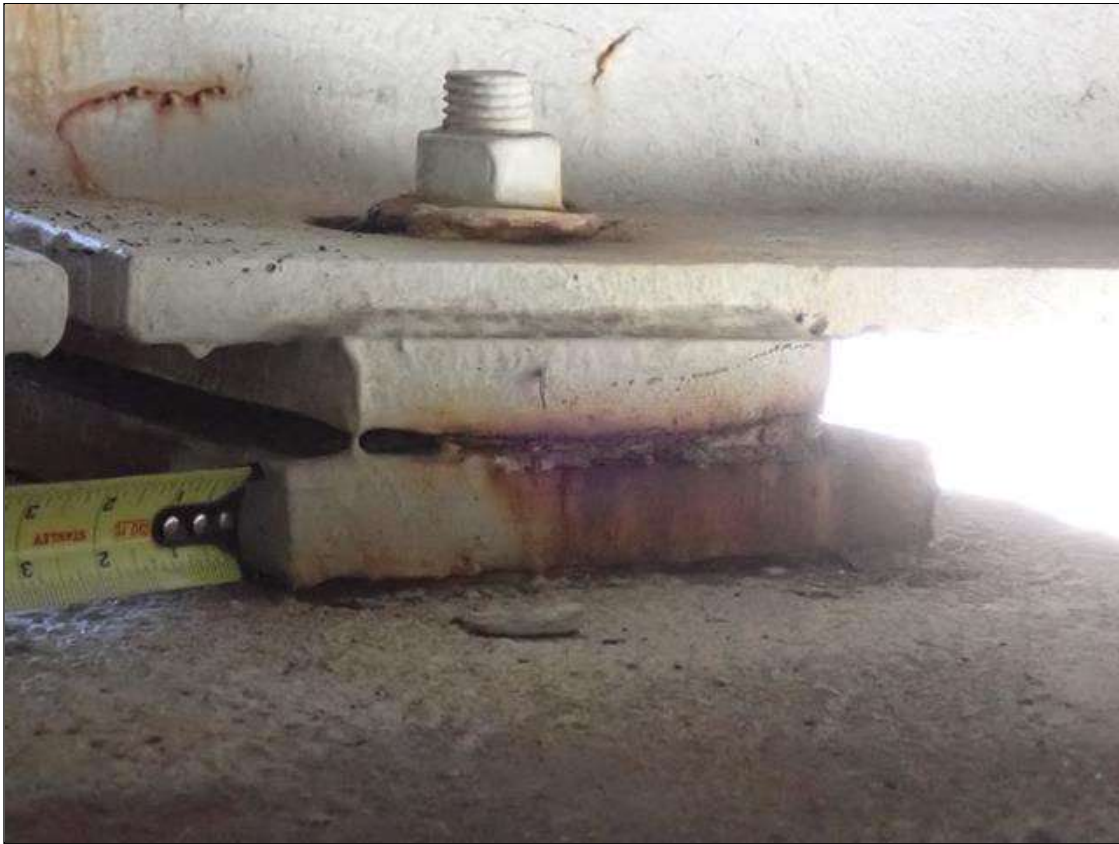
Span 2 Beam 1 - Near Bearing 1: surface rust/pack rust.
