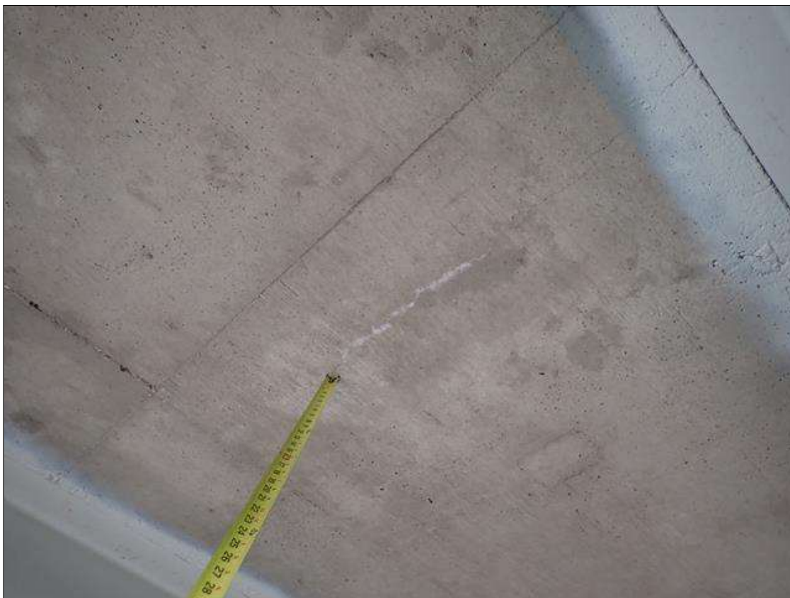
Span 1 Deck: up to 1/32 inch transverse cracks, some with efflorescence, on underside of deck throughout
