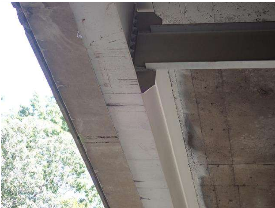
Span 2 Beam 1: underside of bottom flange, over right travel lane, impact scrapes
