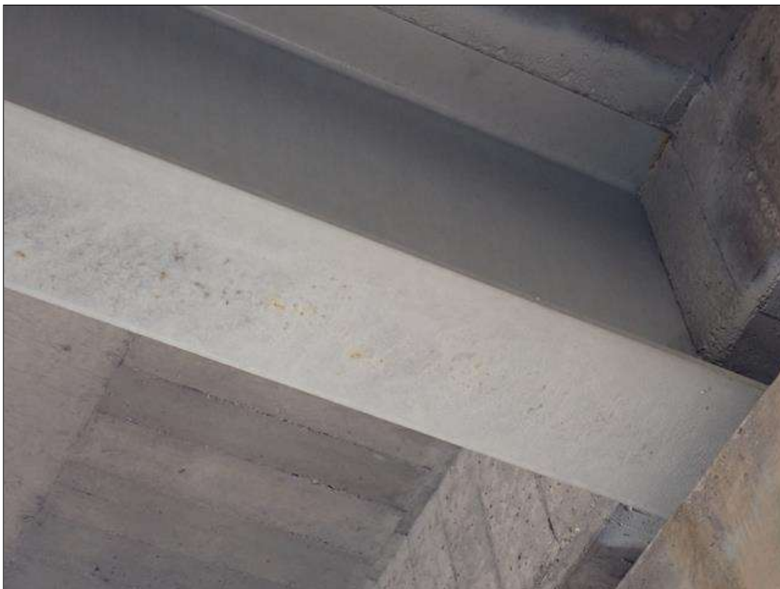
Span 2 Beam 4: underside of bottom flange, near bent 1, freckled rust
