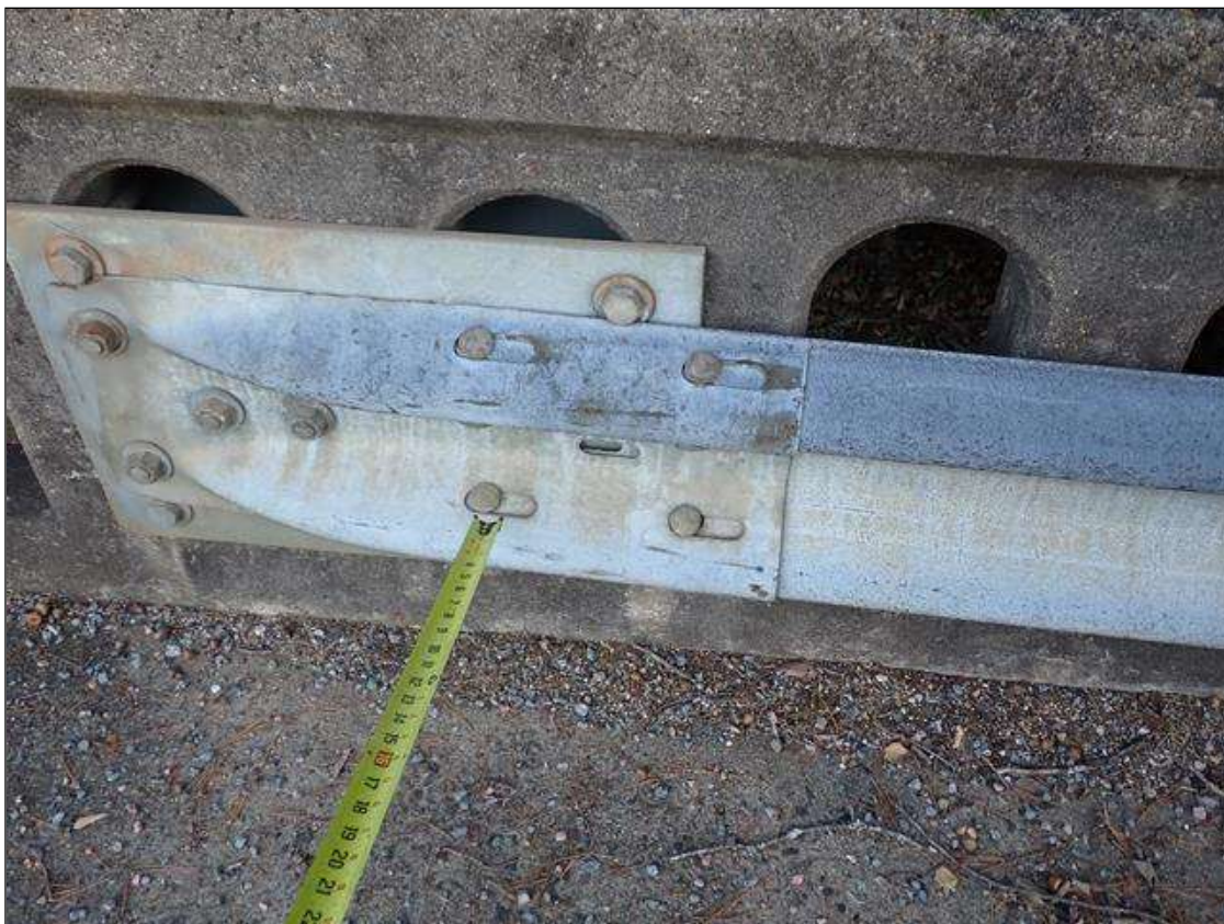
(PAR) northwest guardrail attachment, improper lap
