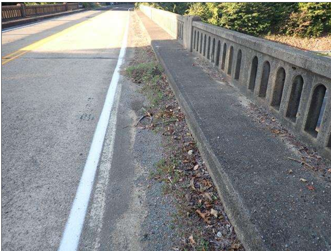
along the curblines, debris accumulation (up to 3.5 feet wide x 10 inches wide) with vegetation, obstructing deck drainage; primarily along left curb
