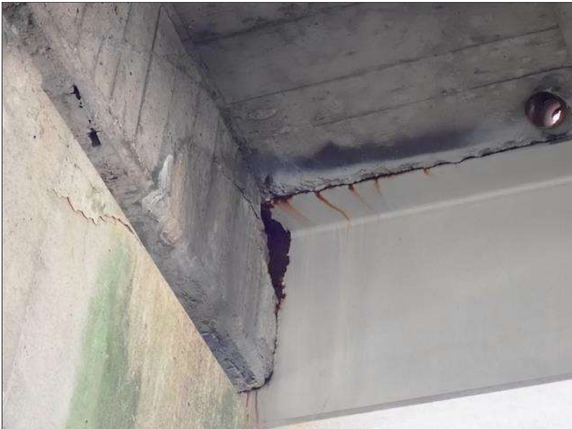
Span 3 Beam 1: at bent 2, web adjacent to diaphragm, painted over pitting (up to 1/8 inch deep x 4 inch x 1 inch) with corrosion reinitiated; web and top flange, surface rust
