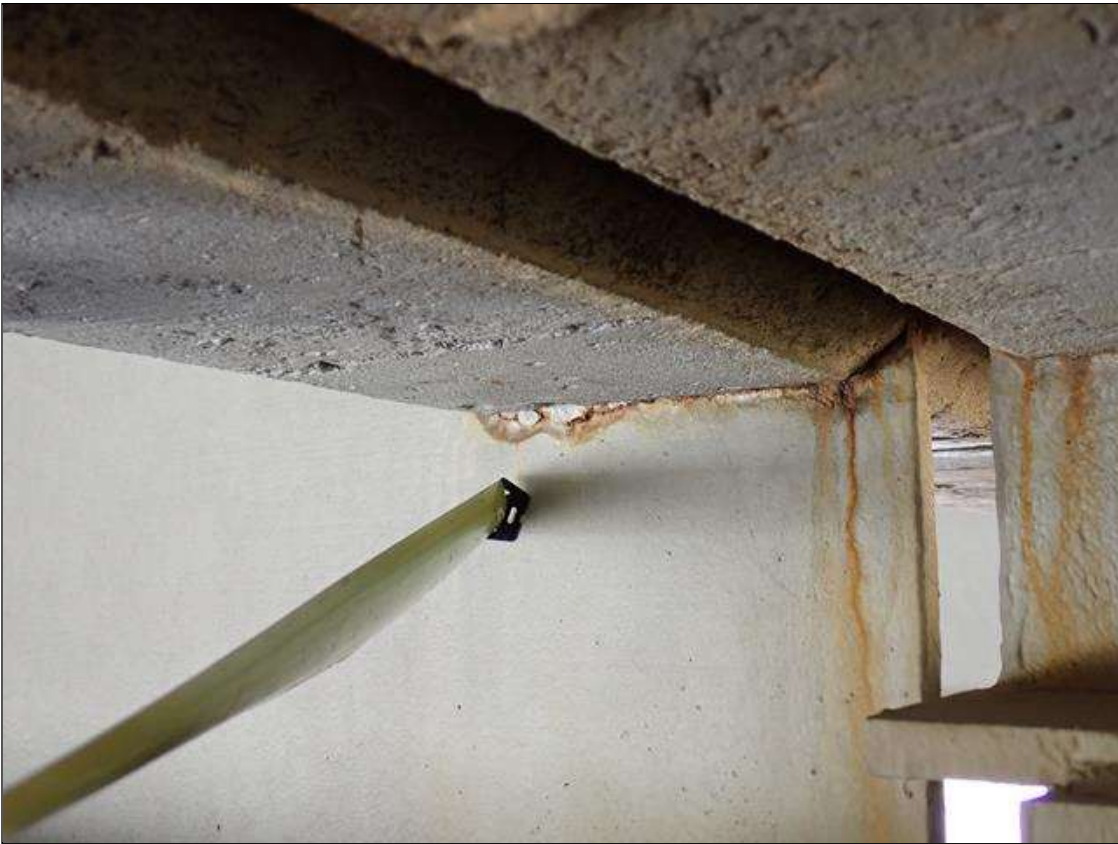
Span 3 Beam 3: (PAR) at bent 3, web adjacent to diaphragm, painted over section loss (3/8 inch average remaining x 9 inch x 1 inch) with corrosion reinitiated
