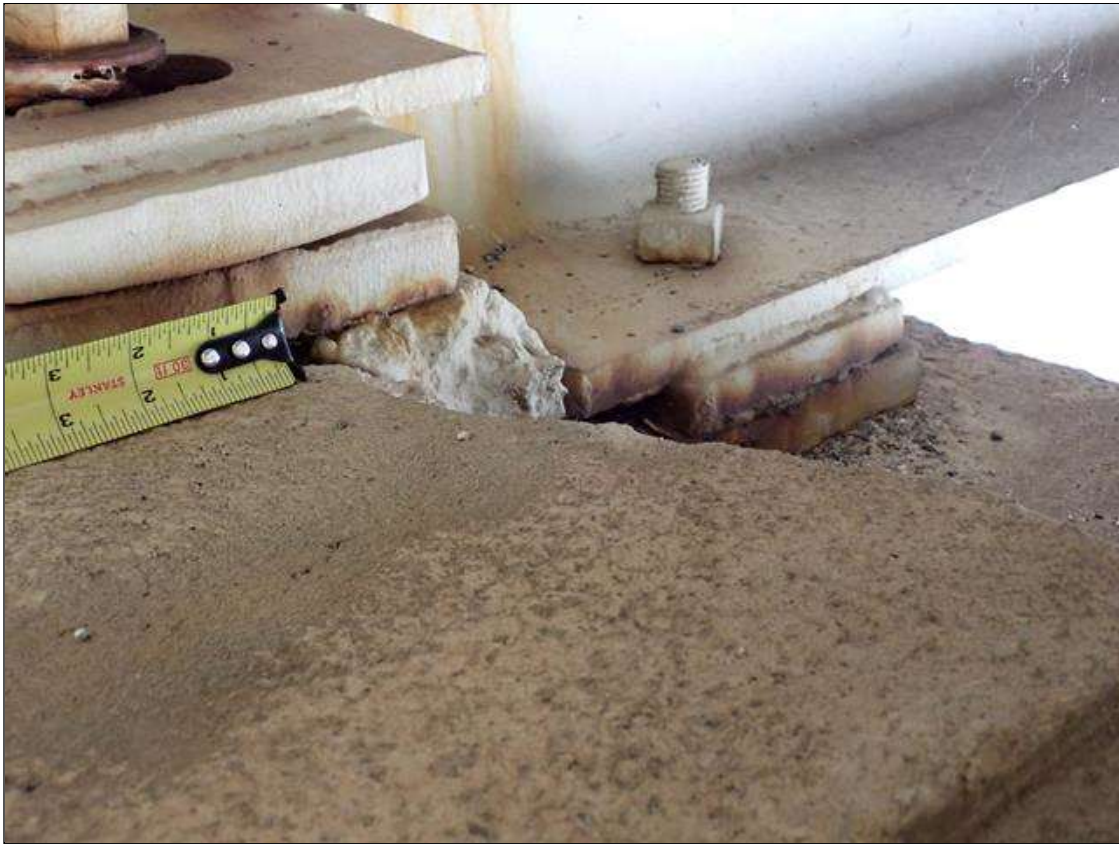
Bent 3 Cap 1: (PAR) at span 4 beam 4 cap step, south face, spall/delamination (2.5 feet x 7 inch x 4 inches deep) undermining bearing
