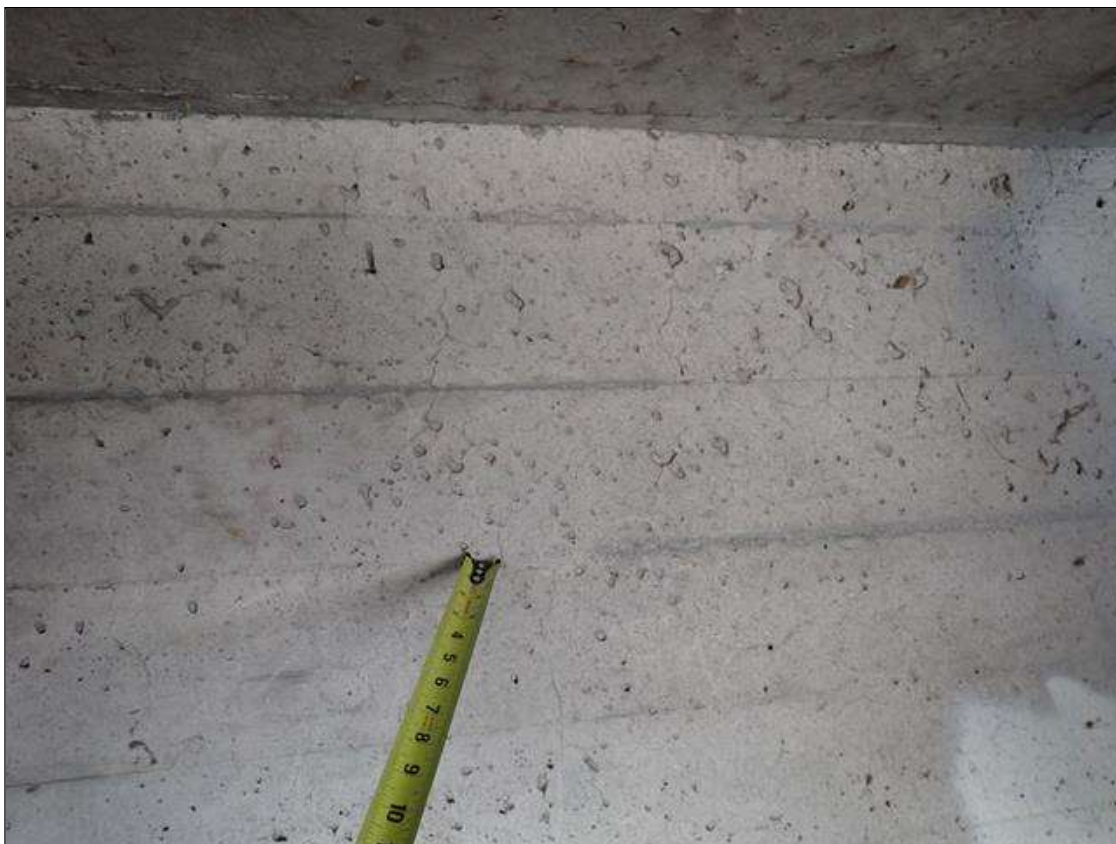
End Bent 2 Abutment: throughout backwall in all bays, multiple areas of hairline map cracking
