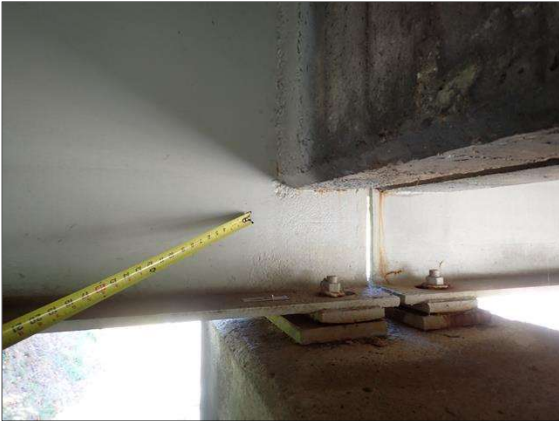
Span 1 Beam 1: (PAR) at bent 1, web adjacent to diaphragm, painted over section loss (3/8 inch average remaining x 3 inch x 2 inch); painted over pitting: lower web (up to 1/8 inch deep x 1 foot x 1 foot); bottom flange (up to 1/8 inch deep x 1 foot); underside of bottom flange, rust scale
