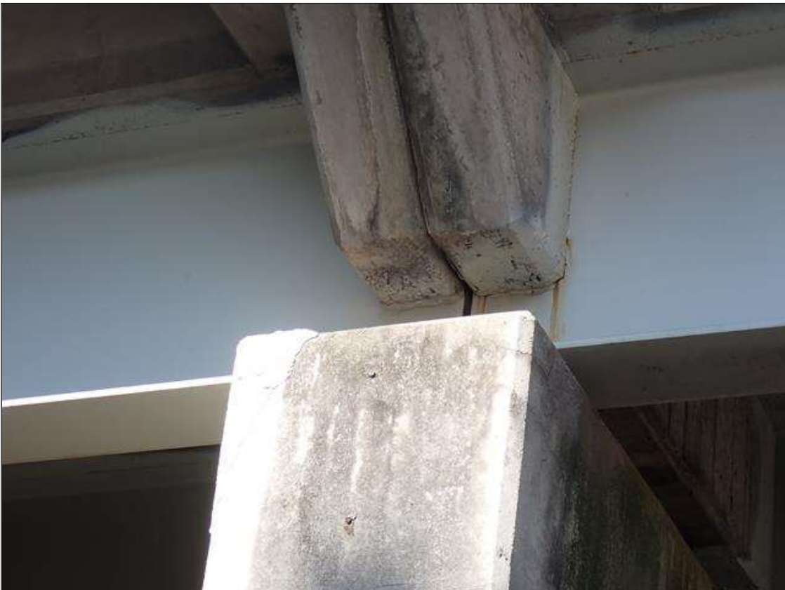
Span 1 Beam 5: (PAR) at bent 1, web adjacent to diaphragm, painted over section loss (approximately 3/8 inch average remaining x 8 inch x 1 inch); no safe ladder access to exterior face
