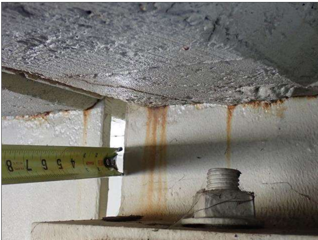
Span 1 Beam 4: at bent 1, web adjacent to diaphragm, painted over section loss (7/16 inch average remaining x 4 inch x 1 inch) with corrosion reinitiated
