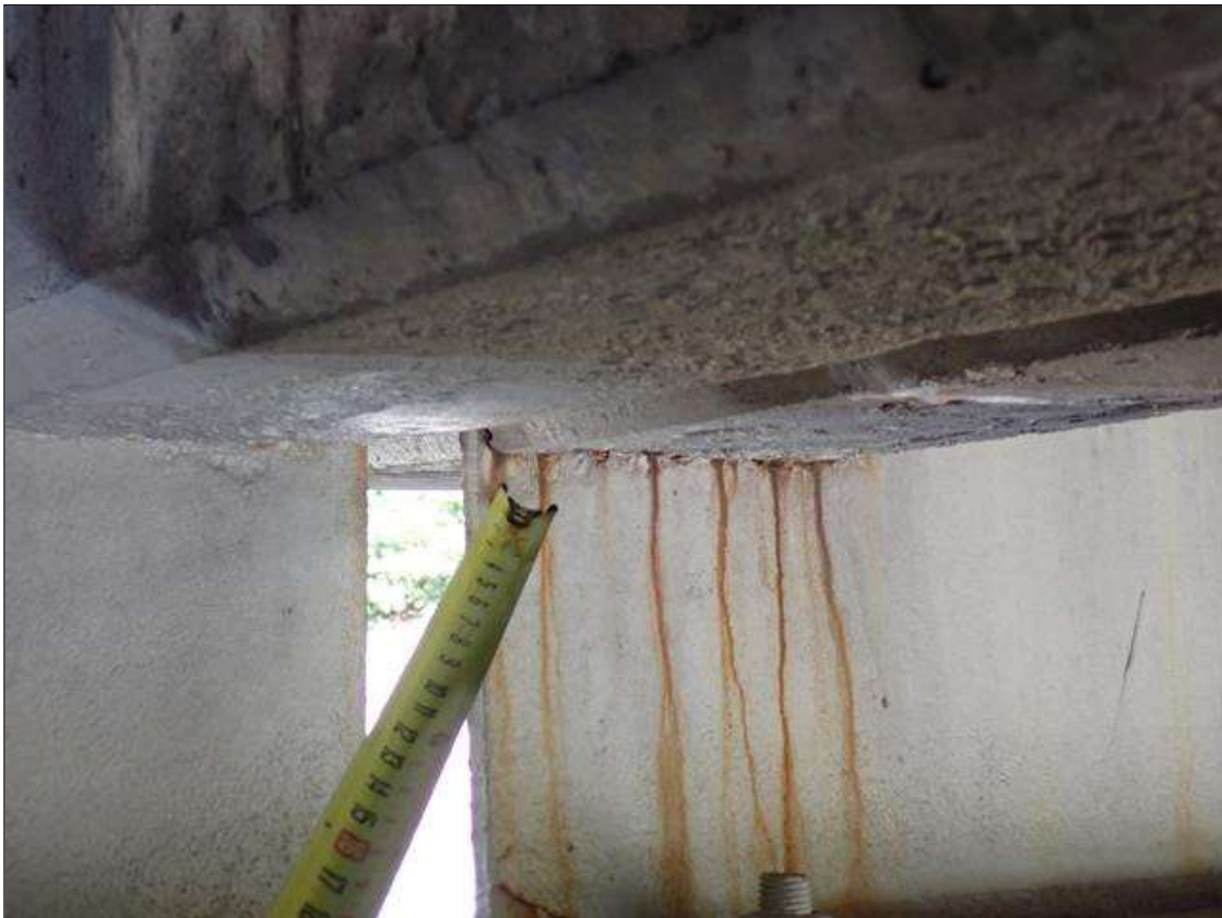
Span 3 Beam 1: at bent 2, web adjacent to diaphragm, painted over pitting (up to 1/8 inch deep x 4 inch x 1 inch) with corrosion reinitiated; web and top flange, surface rust
