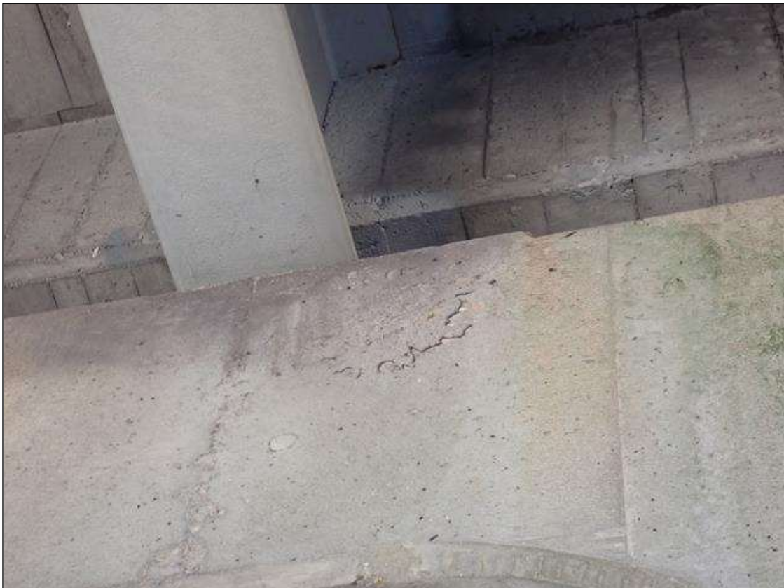
Bent 1 Cap 1: at North face under beam 2, delamination [1 foot diameter]
