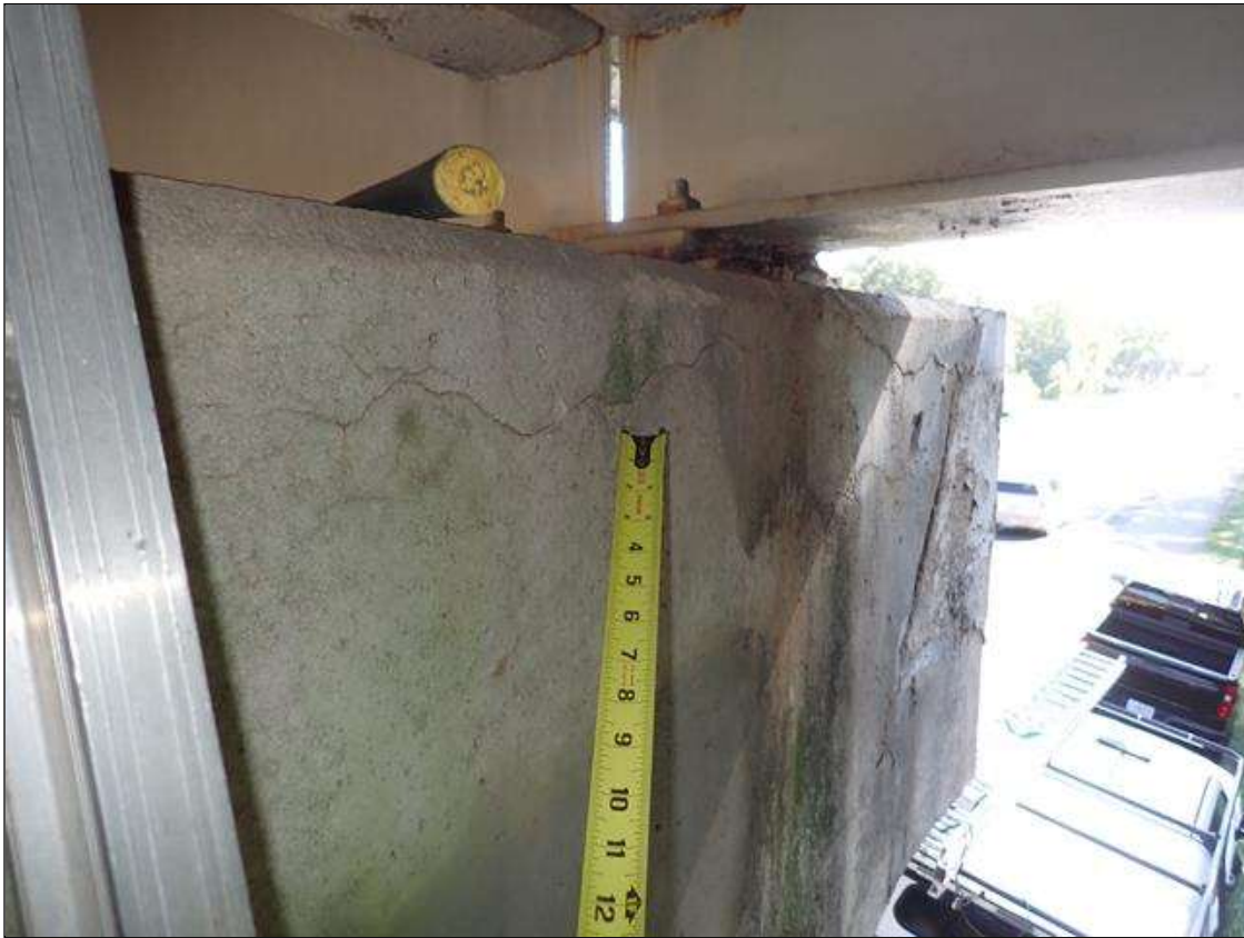
Bent 1 Cap 1: south face, below bay 4 and right overhang, along top edge, delamination (6 feet x 8 inch) with associated cracks (up to 1/32 inch); southeast corner, patched area (20 inch x 18 inch)
