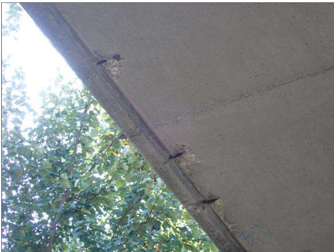
Span 1 Deck: (PAR) 7 - spalls with exposed reinforcing up to 4 inch diameter x 1 inch deep, in underside of right overhang, at random.
