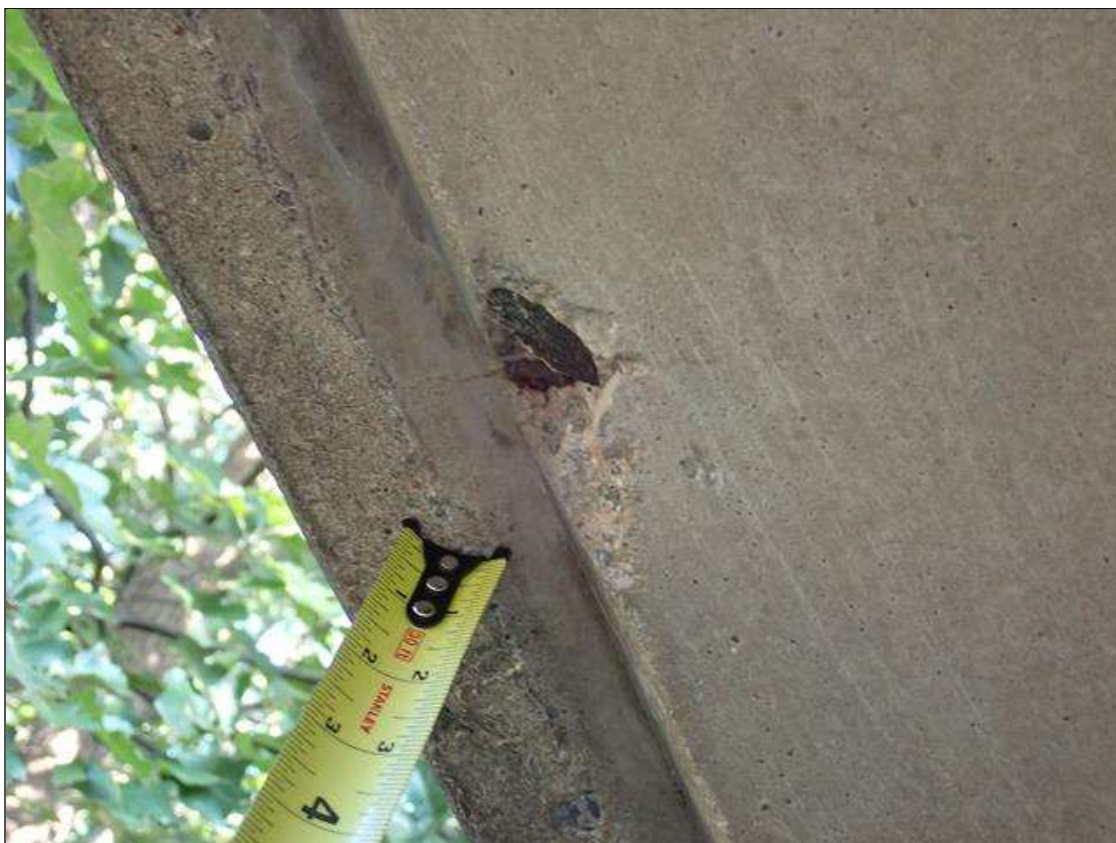
Span 4 Deck: (PAR) 5 - spalls with exposed reinforcing up to 4 inch x 2 inch x 1 inch deep, in underside of left overhang, at random.
