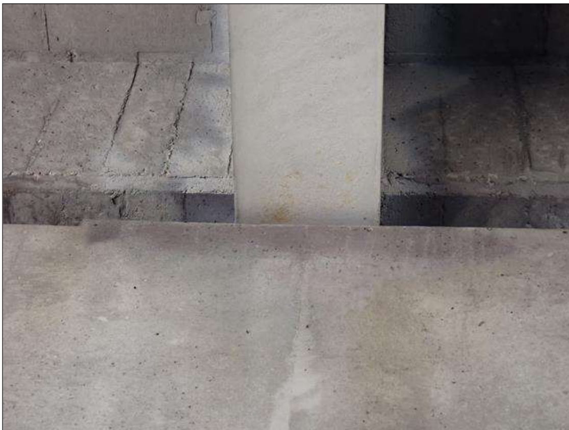
Bent 2 Cap 1: (not found 2023) under beam 4, delamination [1 foot x 1.5 feet]
