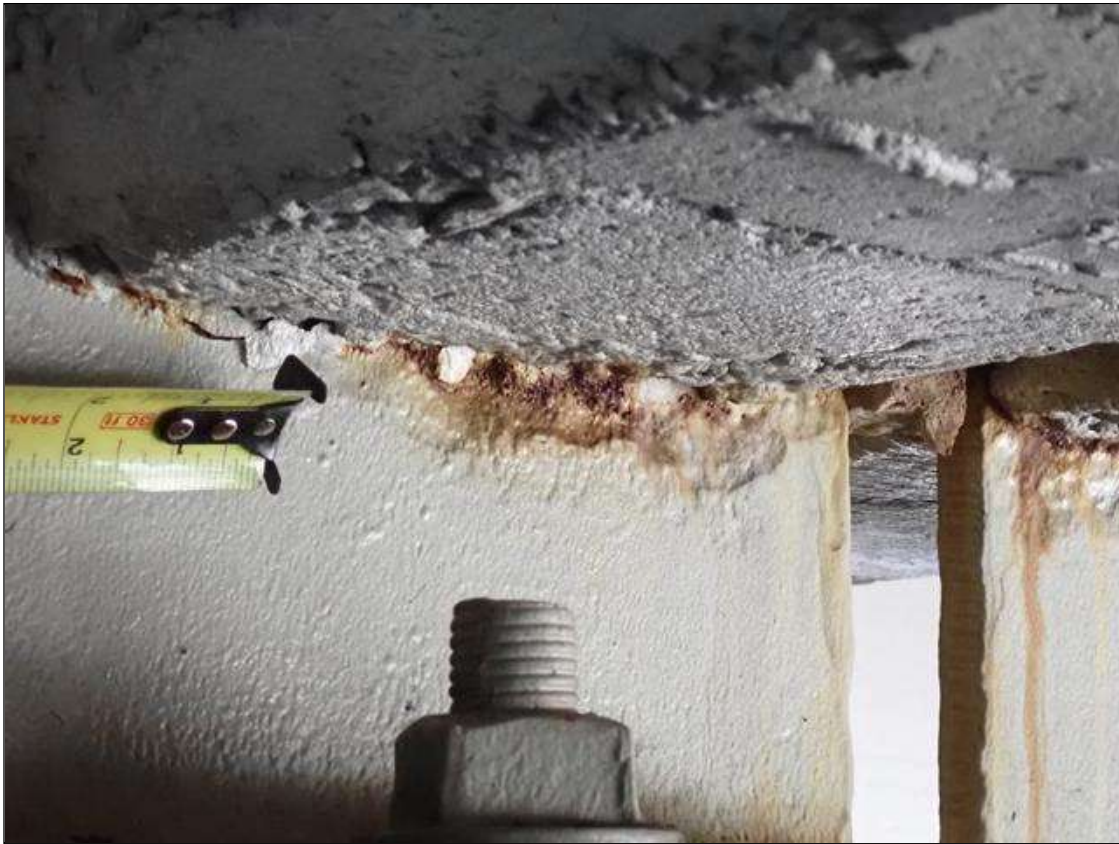
Span 1 Beam 3: (PAR) at bent 1, web adjacent to diaphragm, painted over section loss (5/16 inch average remaining x 6 inch x up to 2 inch) with corrosion reinitiated
