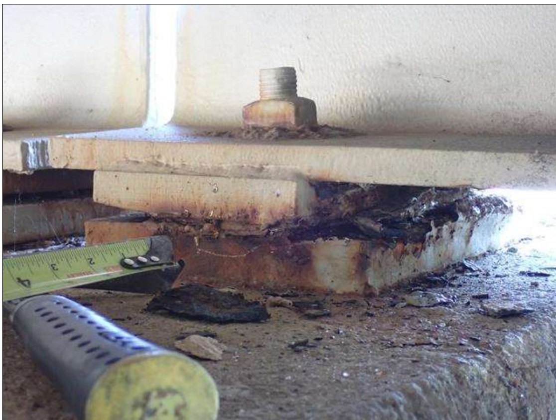
Span 1 Beam 5 - Far Bearing 5: corrosion with section loss (up to 1/8 inch deep) and pack rust
