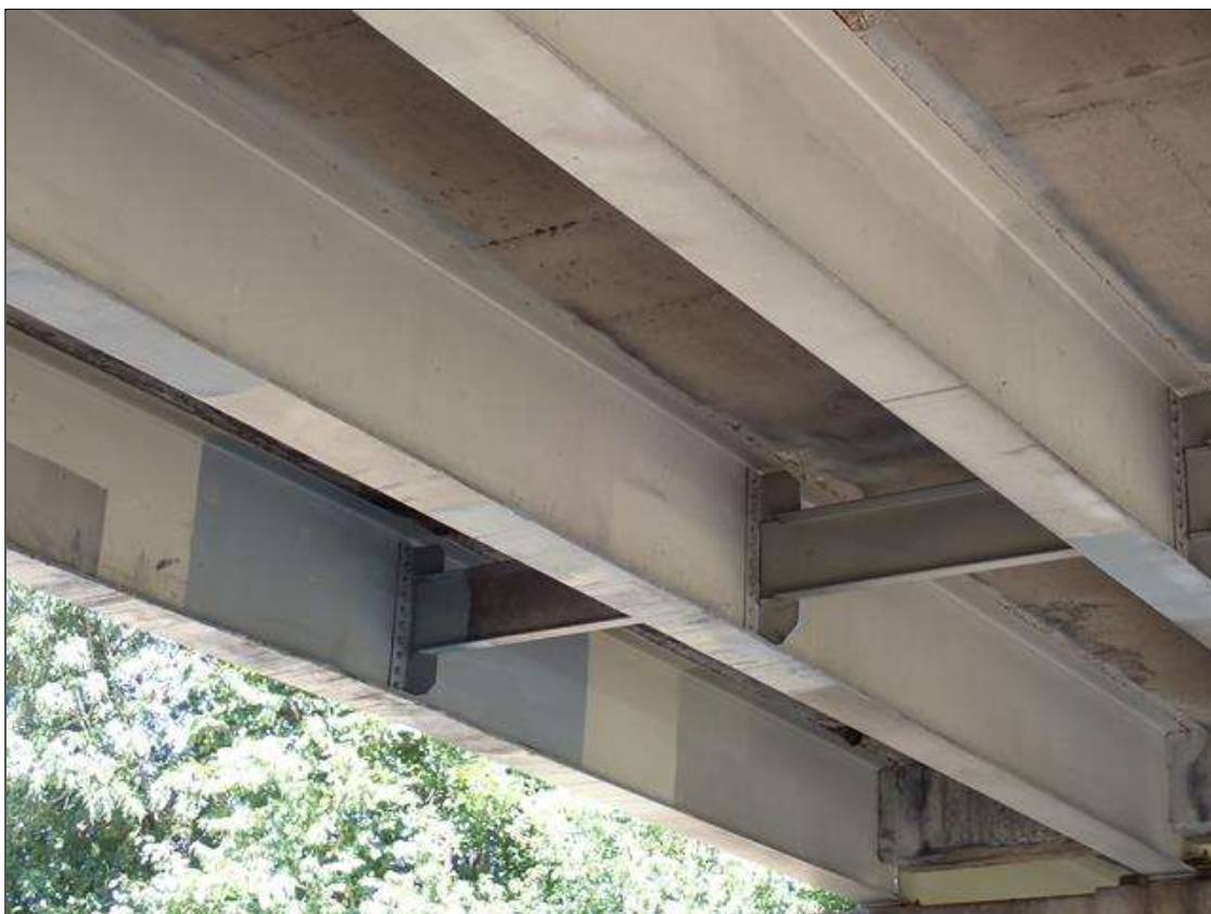
Span 3 Beam 2: (not found 2023) SUPPLEMENTAL INSPECTION IMPACT DAMAGE 2022.: SCATTERED SCRAPES WEB OF BEAM 2 .
