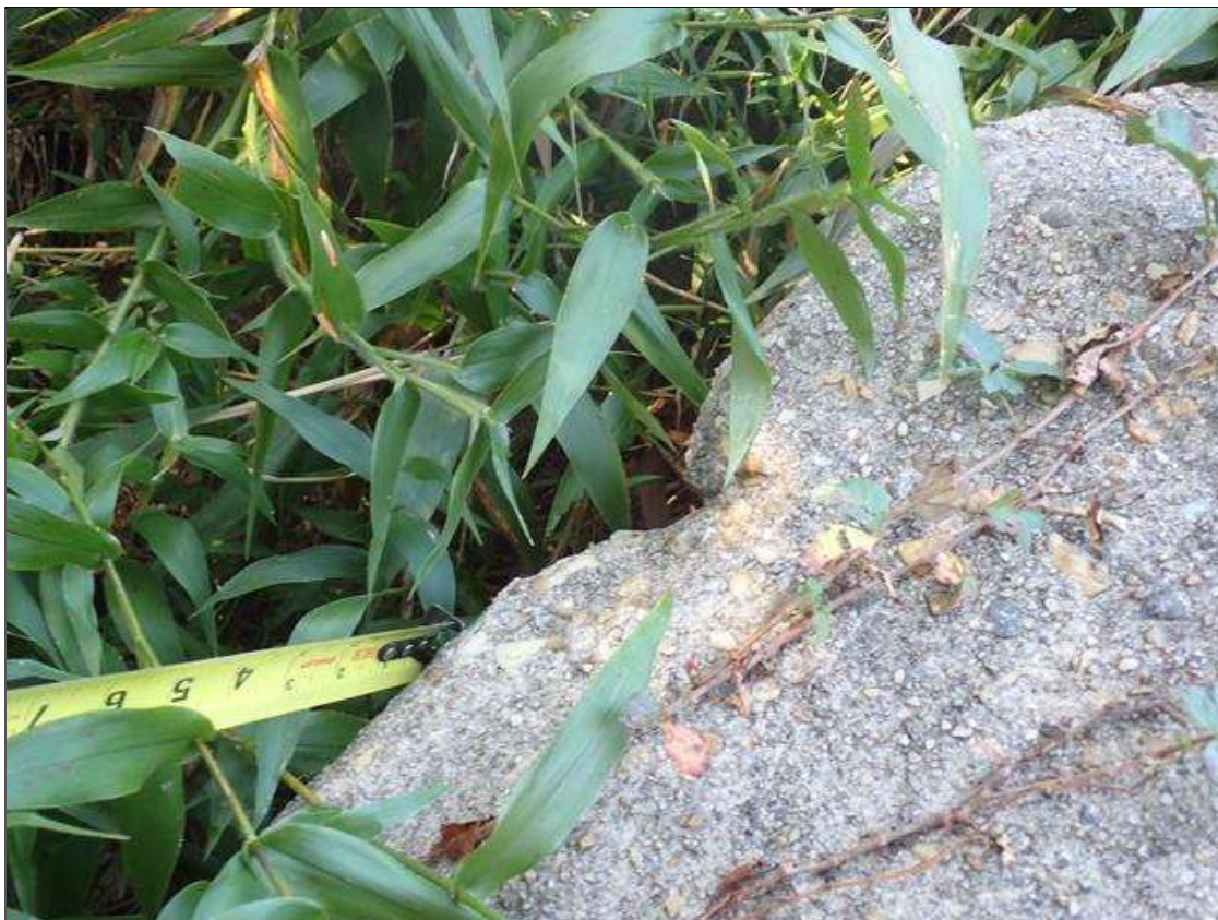
southeast wingwall, along top, spall (6 inch diameter x 1.5 inch deep)
