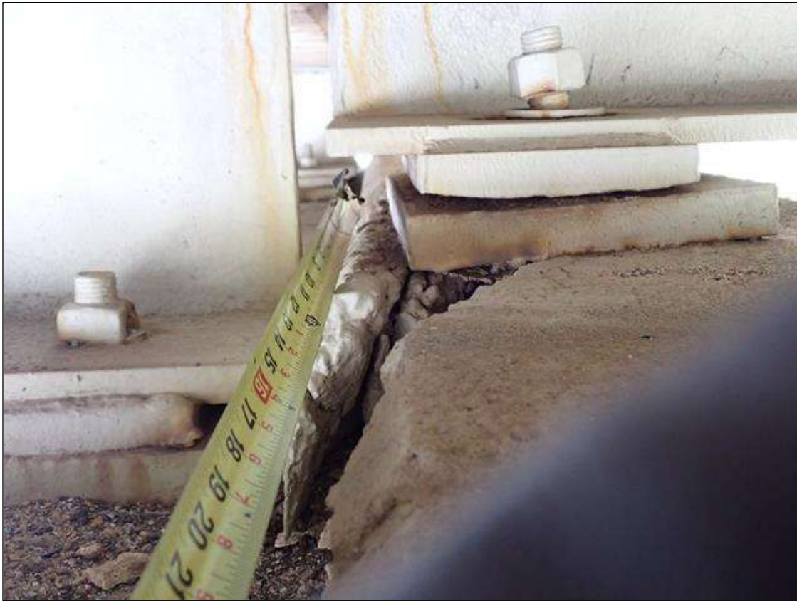
Span 4 Beam 3 - Near Bearing 3: (PAR) south edge of masonry plate, undermined (13 inch x 3 inches deep) due to cap step spall; masonry plate displaced downward (up to 1/2 inch)
