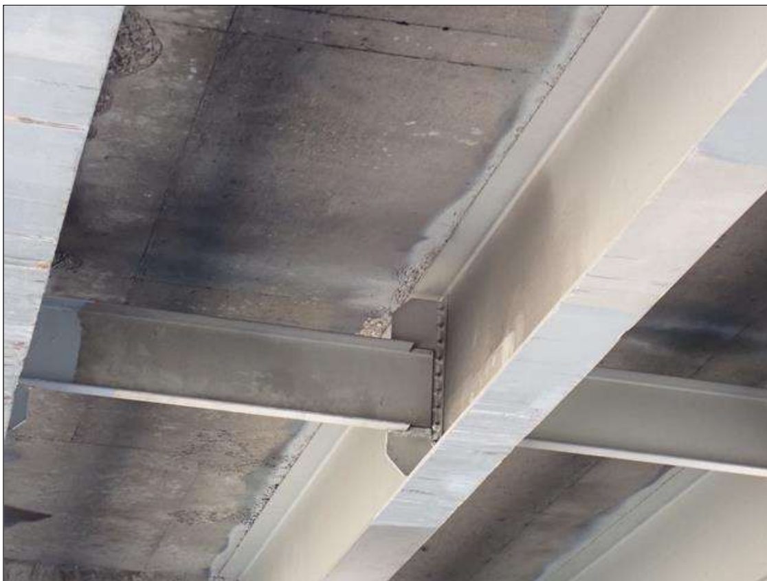
Span 3 Deck: surface spalling up to 1 foot x 4 inch x 1/2 inch deep, full length, underside of deck along both sides of beam 2.
