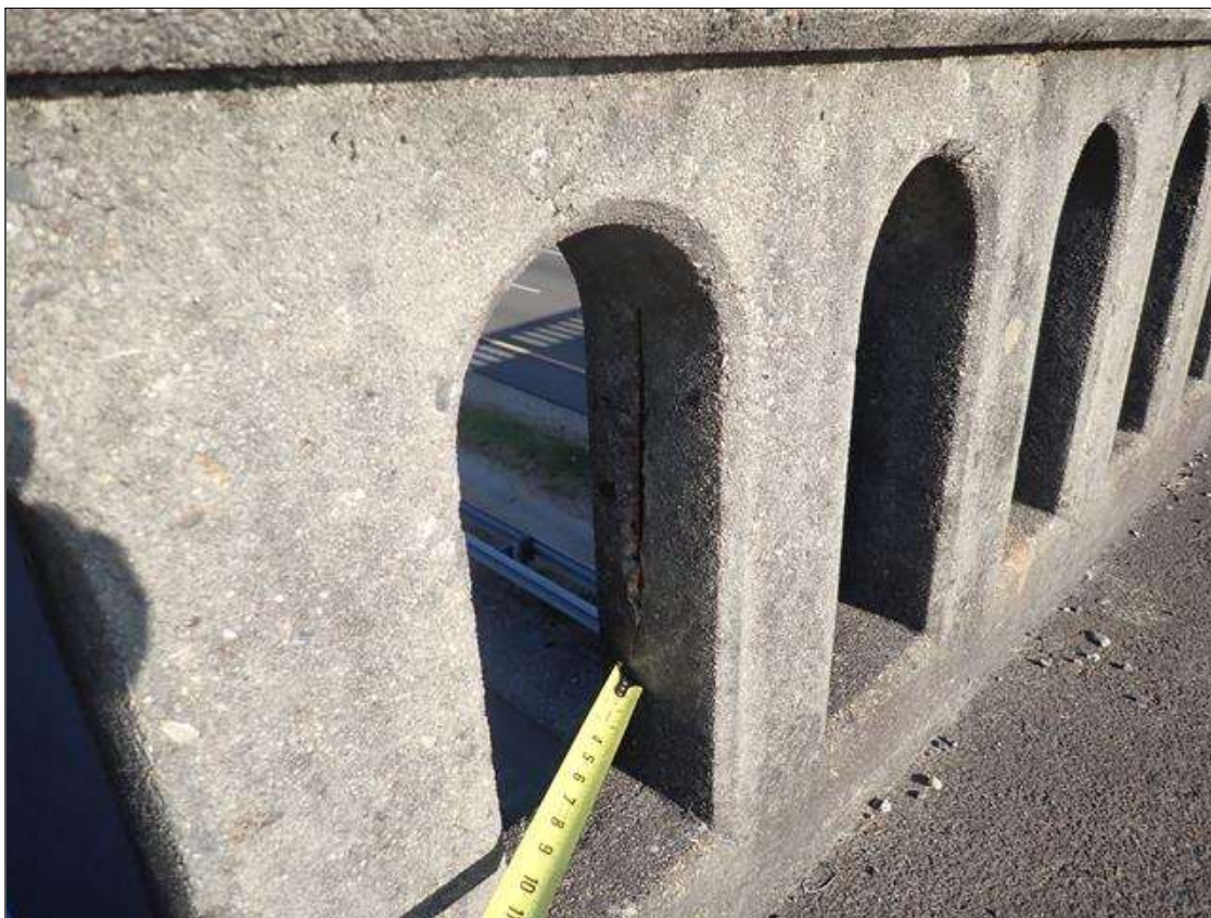
Span 2 Left Bridge Rail: 6 - spalls with exposed reinforcing up to 8 inch x 1 inch x 1/2 inch deep, at random.
