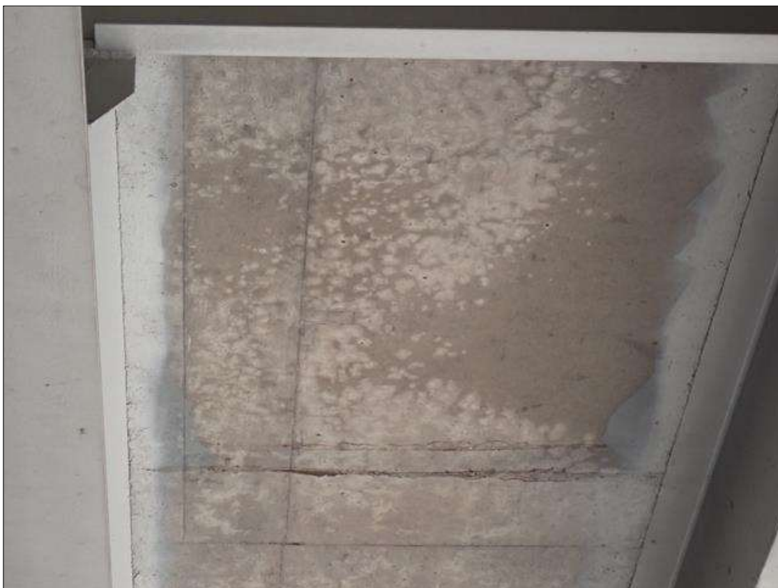
Span 2 Deck: throughout underside in all bays, multiple areas of hairline map cracking
