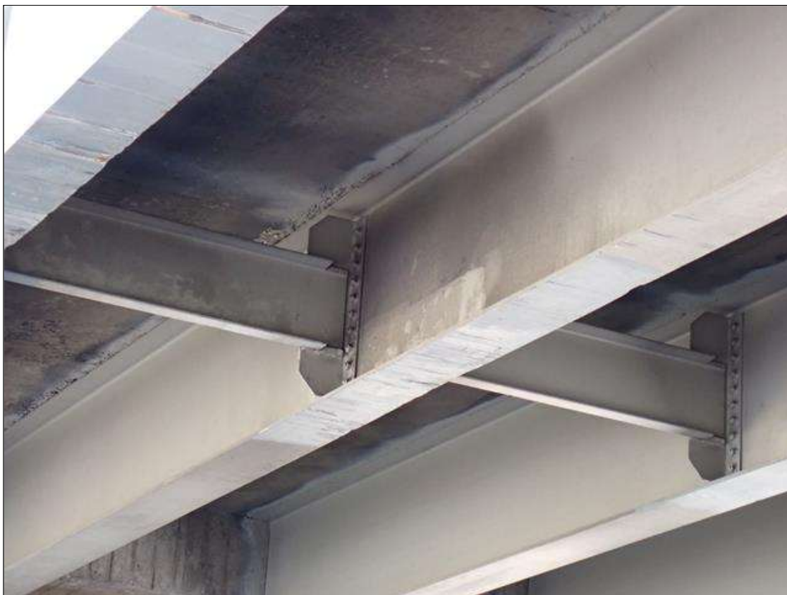
Span 3 Beam 2: (not found 2023) SUPPLEMENTAL INSPECTION IMPACT DAMAGE 2022.: SCATTERED SCRAPES WEB OF BEAM 2 .
