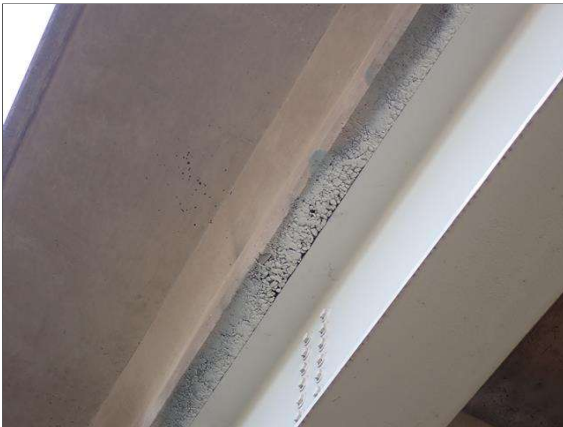
Span 1 Deck: throughout underside of deck, scattered areas of poor consolidation (up to 1/2 inch deep) at random
