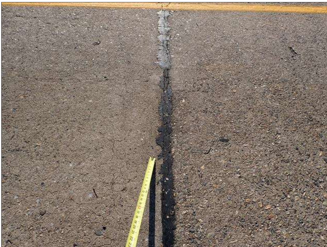
Span 3 Expansion Joint at Bent 2: along the length of the joint, seal cracks at random
