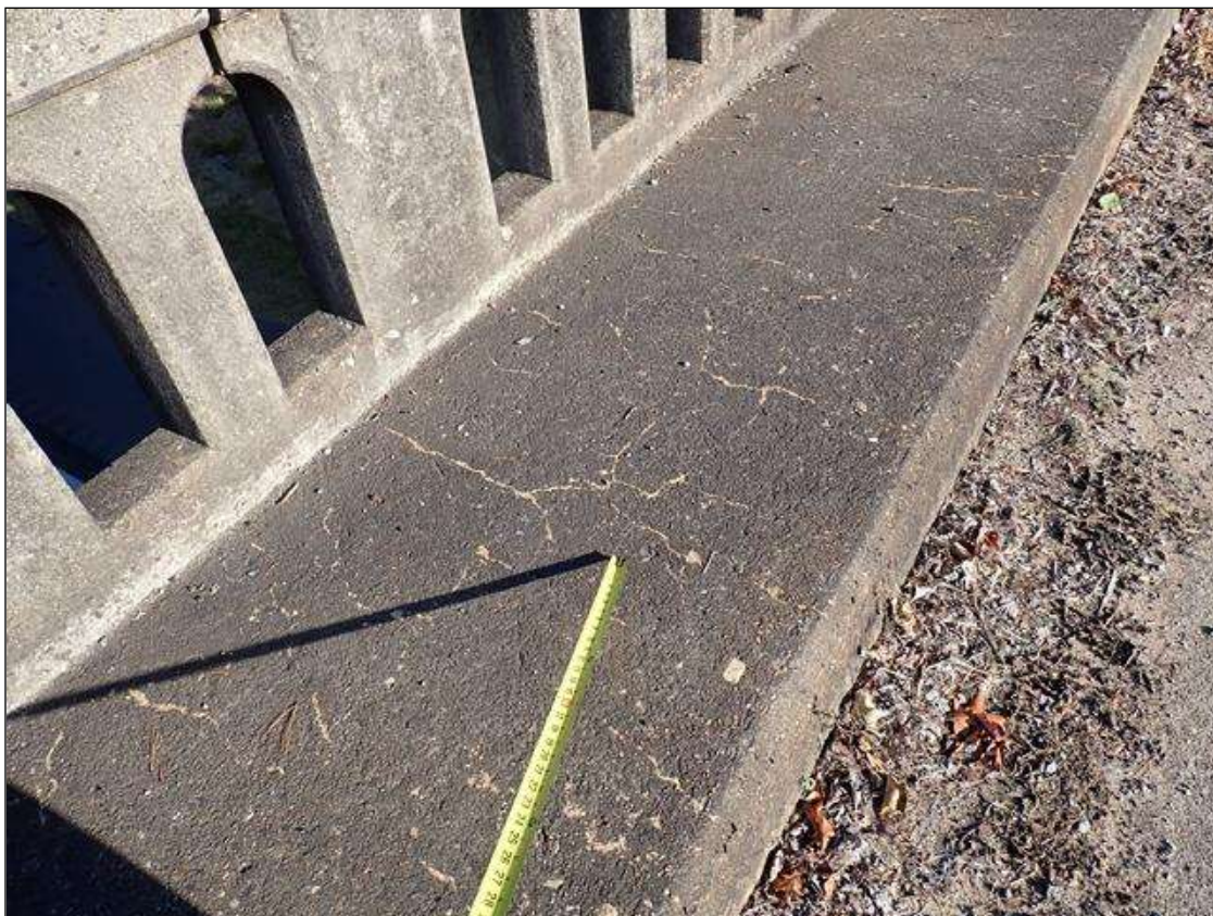
Span 3 Deck: throughout left sidewalk, multiple areas hairline map cracking
