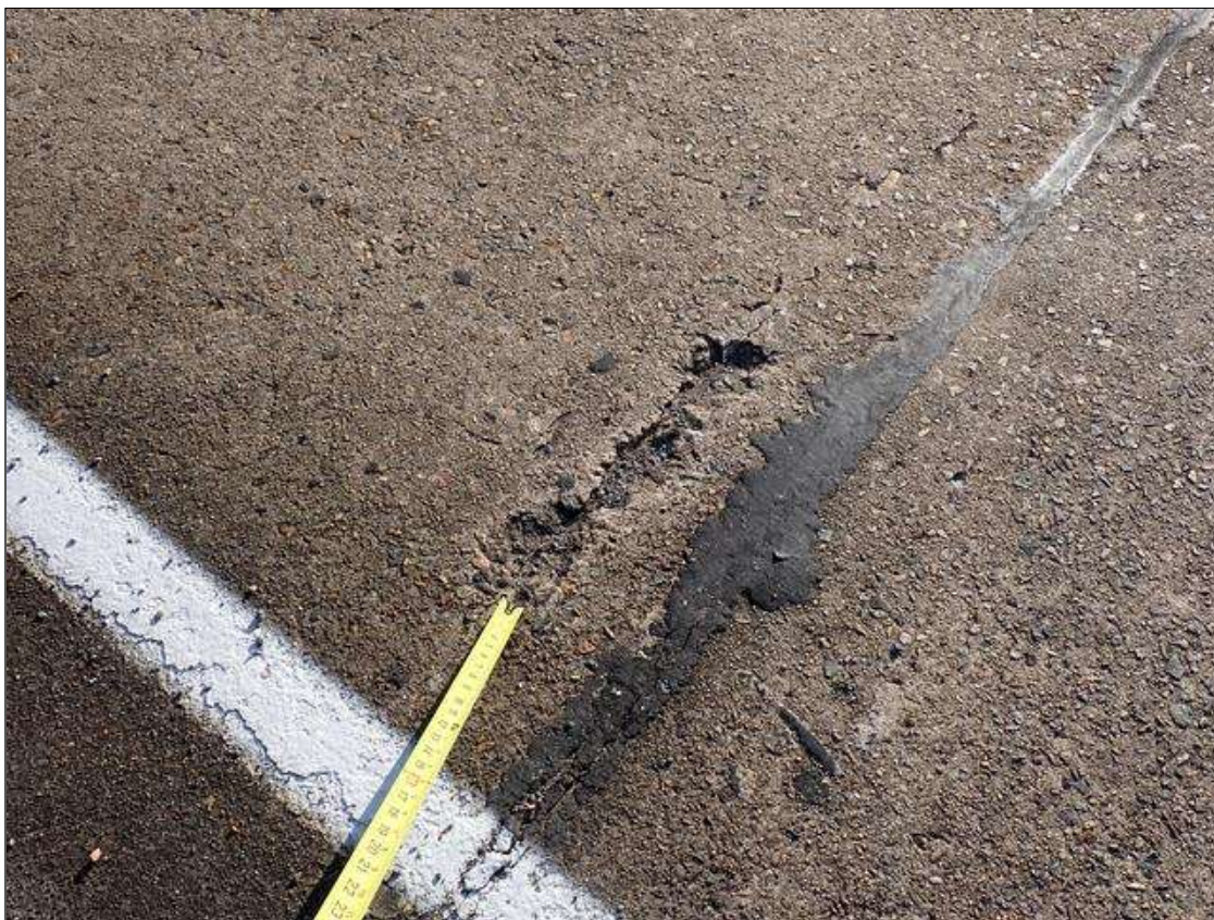
Span 2 Deck: (PAR) southbound lane, at bent 1, spall (2 feet x 6 inch x 1 inch deep) with exposed rusted rebar
