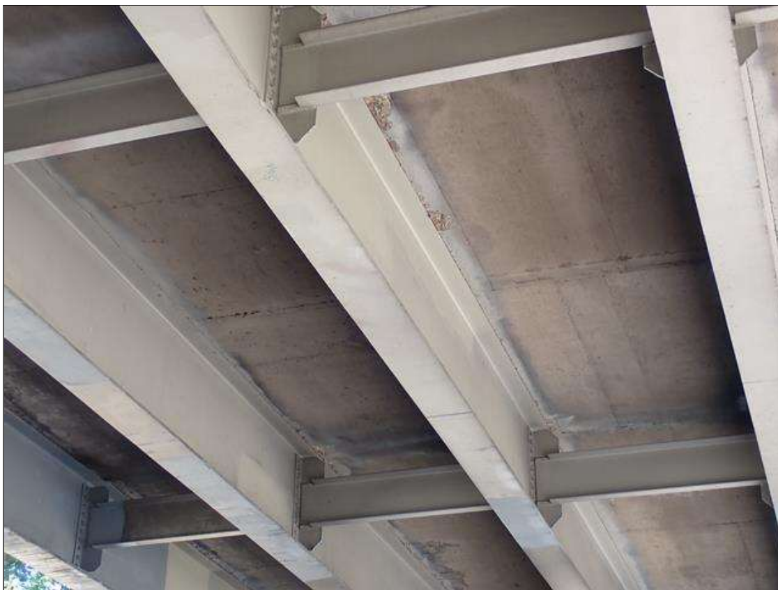
Span 3 Beam 3: beam 3 span 3 deflected upward 1/4 inch for a length of 3 feet at 15 feet from bent 2
