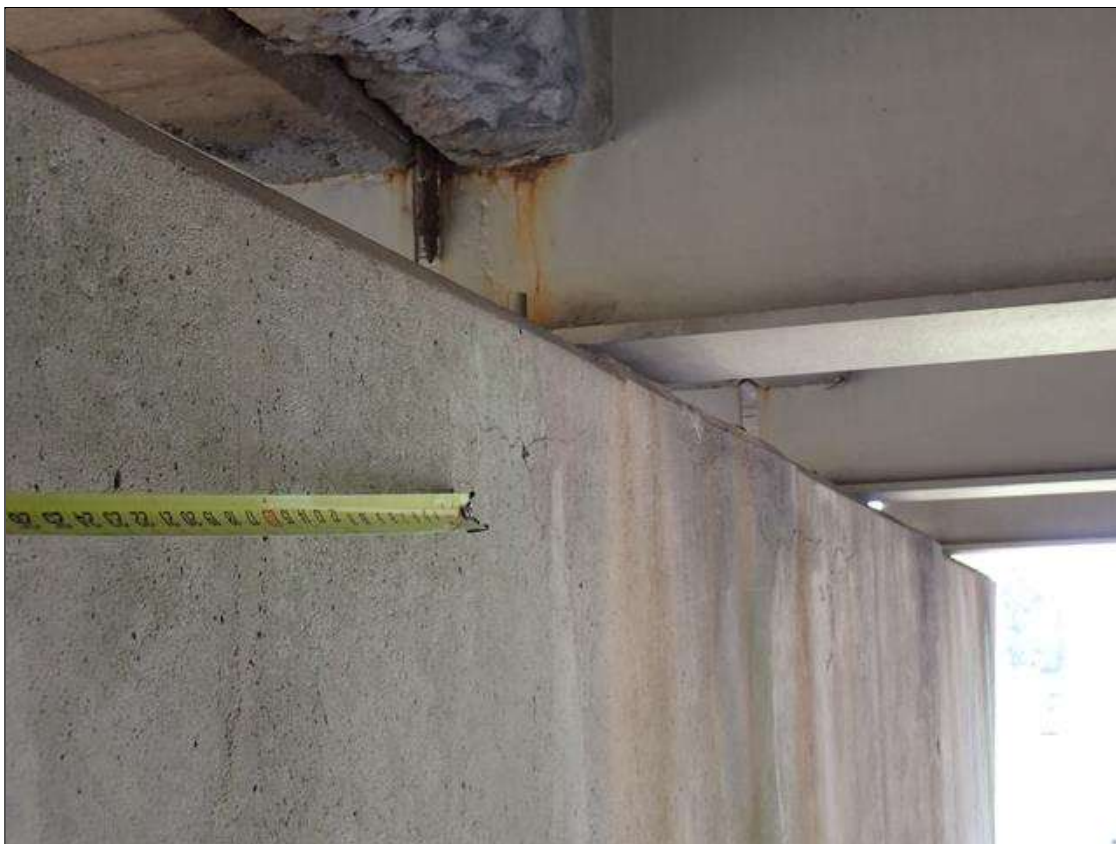
Bent 2 Cap 1: south face, below bays 1-3, longitudinal cracks (up to 1/32 inch x 5 feet) with adjacent map cracks (hairline)
