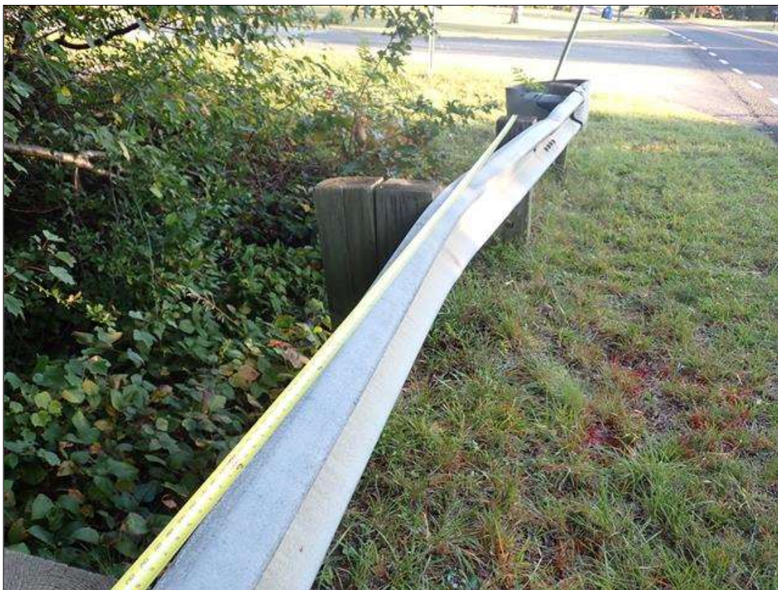
(PAR) northwest guardrail, near termination, impact damage (10 feet)
