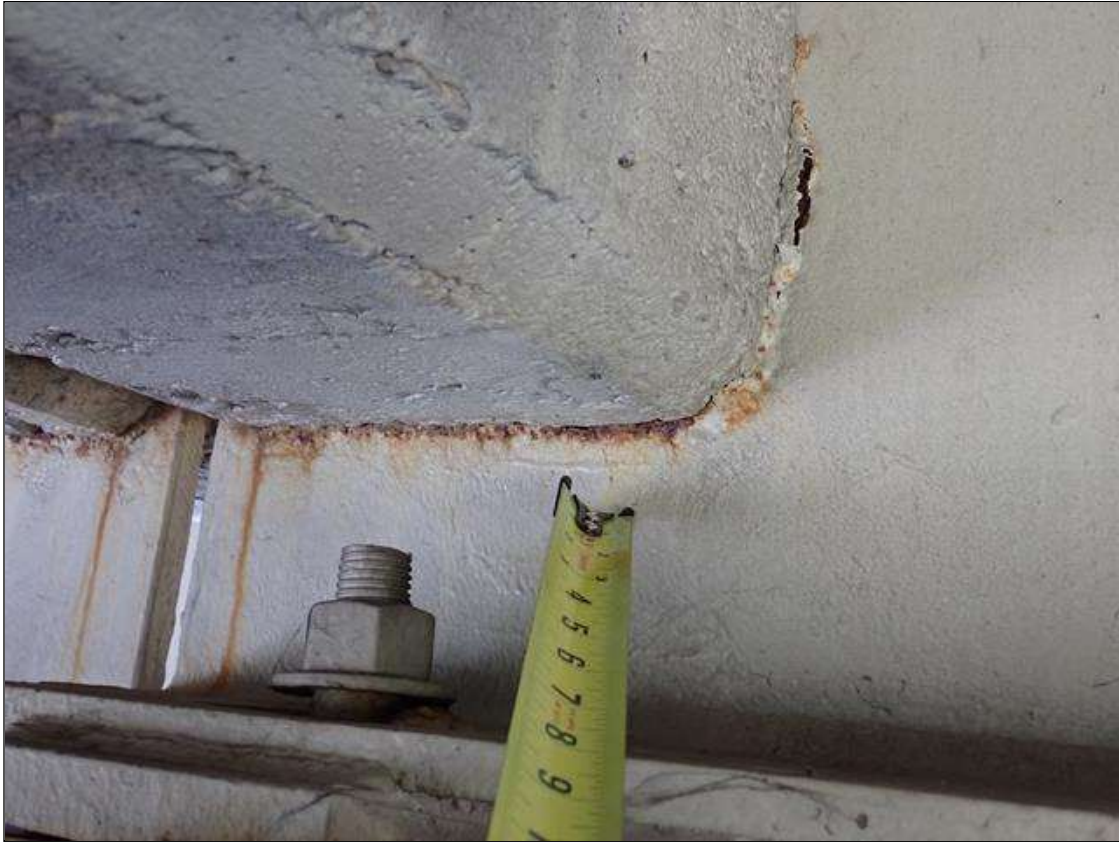
Span 4 Beam 4: at bent 3, web adjacent to diaphragm, painted over section loss (7/16 inch average remaining x 11 inch x 1 inch) with corrosion reinitiated
