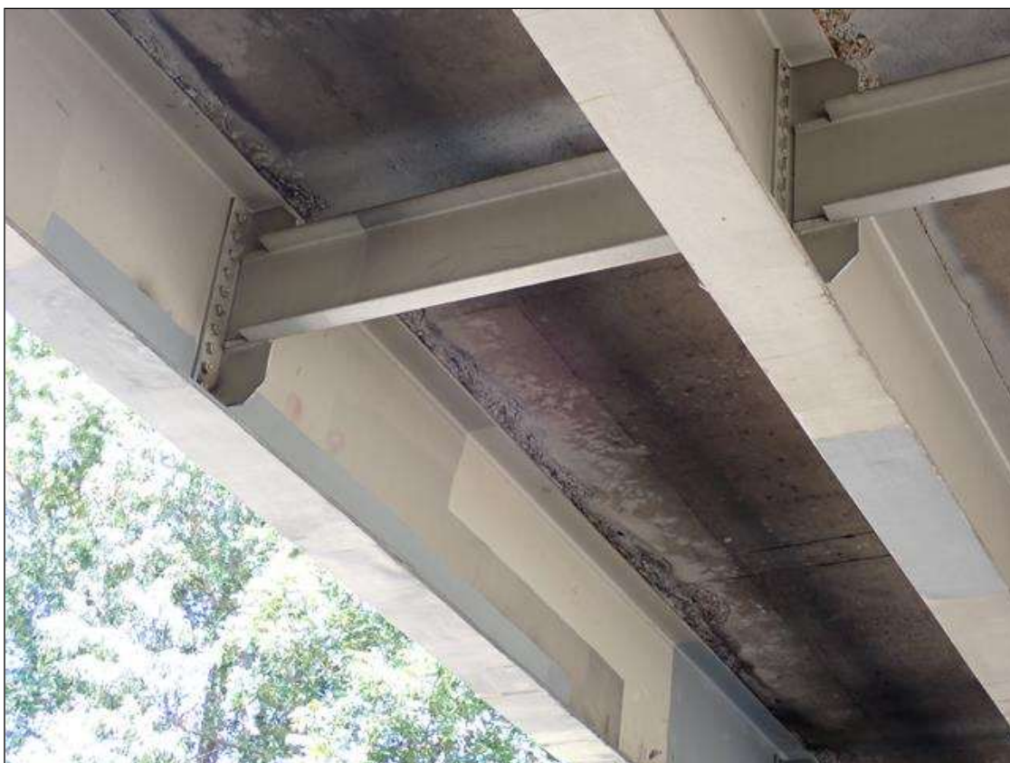
Span 3 Deck: spalling up to 12 INCH WIDE X 1 INCH deep, full length, underside of deck along both sides of beam 1.
