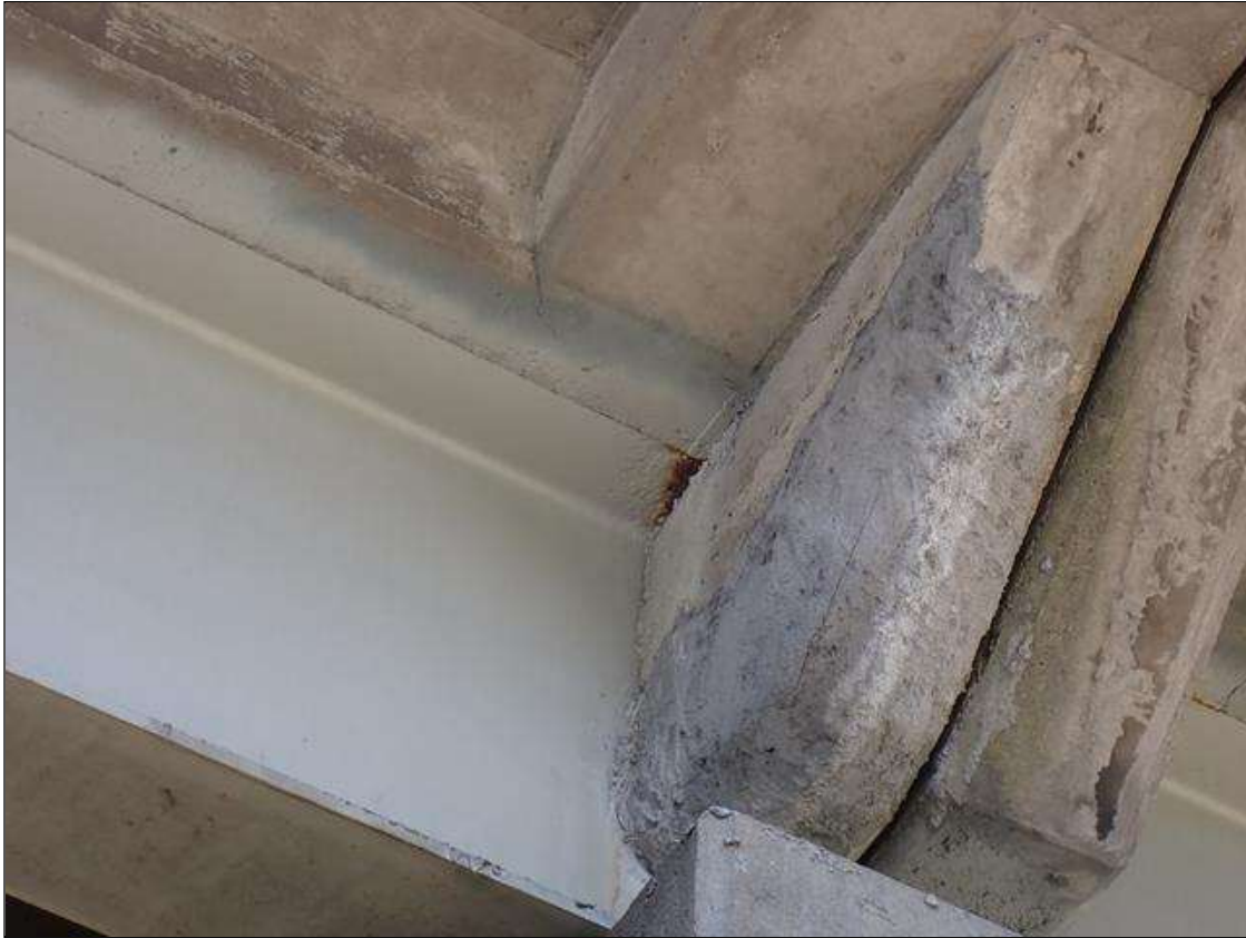
Span 2 Beam 5: (PAR) at bent 2, web adjacent to diaphragm, painted over section loss (3/8 inch average remaining x 9 inch x 1 inch); east top flange, painted over pitting (up to 1/8 inch deep x 6 inches x 4 inches) with corrosion reinitiated
