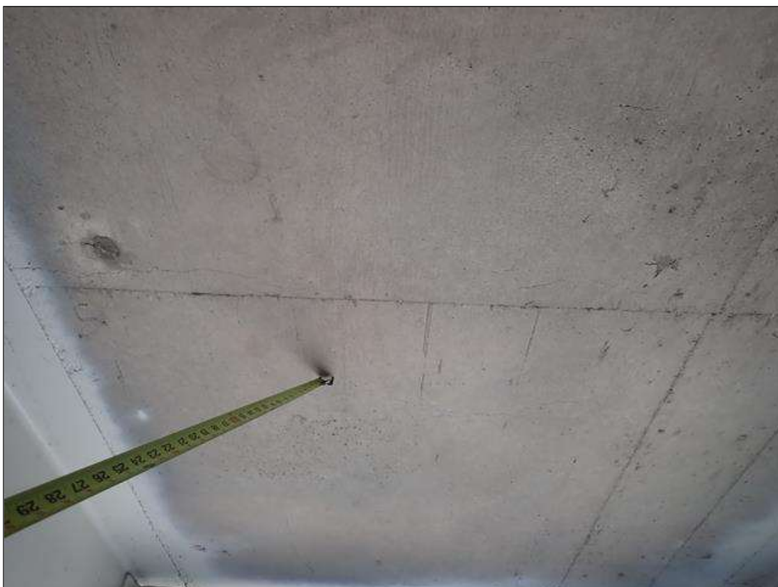
Span 4 Deck: random hairline map cracking and transverse cracks up to 1/32 inch wide on topside and underside.
