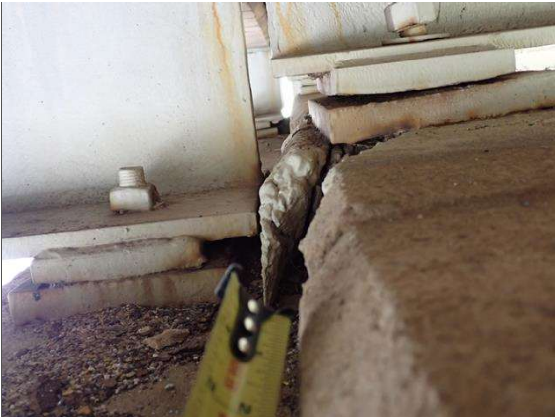
Bent 3 Cap 1: (PAR) at span 4 beam 4 cap step, south face, spall/delamination (2.5 feet x 7 inch x 4 inches deep) undermining bearing
