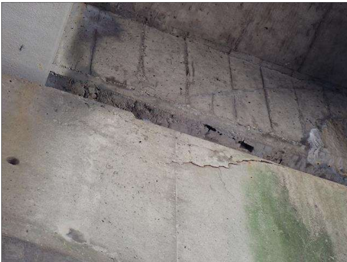
Bent 2 Cap 1: delamination [19 inch x 7 inch] at north face extending to topside, under bay 1.
