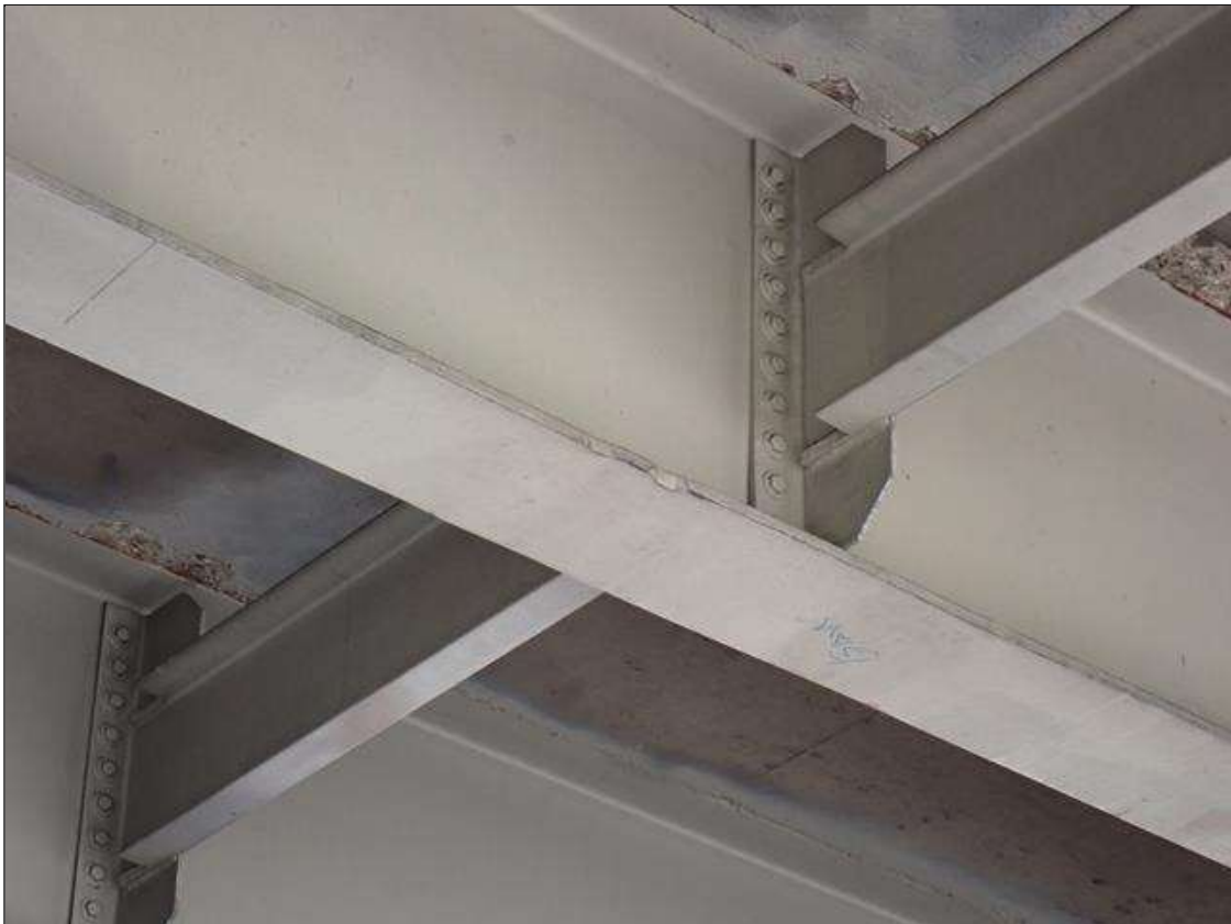
Span 3 Beam 3: two indentions in bottom flange of beam 3 span 3. one 1/4 inch deep and one 1/2 inch deep at 15.583 feet from bent 2 for a total length of 1 foot
