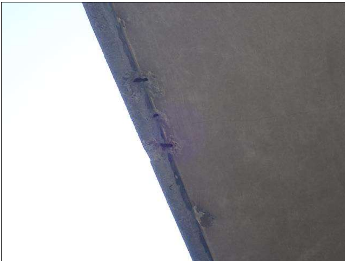
Span 1 Deck: (PAR) 5 - spalls with exposed reinforcing up to 4 inch diameter x 1 inch deep, in underside of left overhang, at random.
