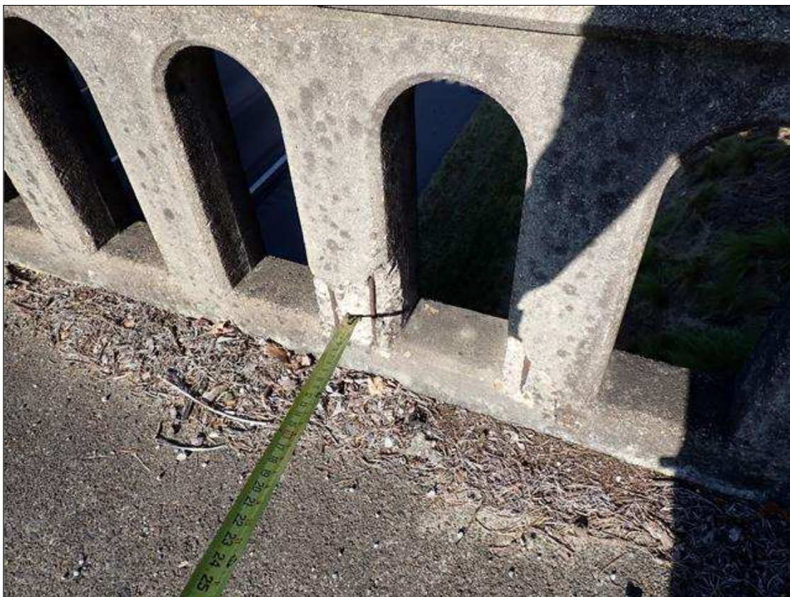
Span 4 Left Bridge Rail: along the length of the rail, spalls (up to 8 inch x 7 inch x 1 inch deep) with exposed rusted rebar
