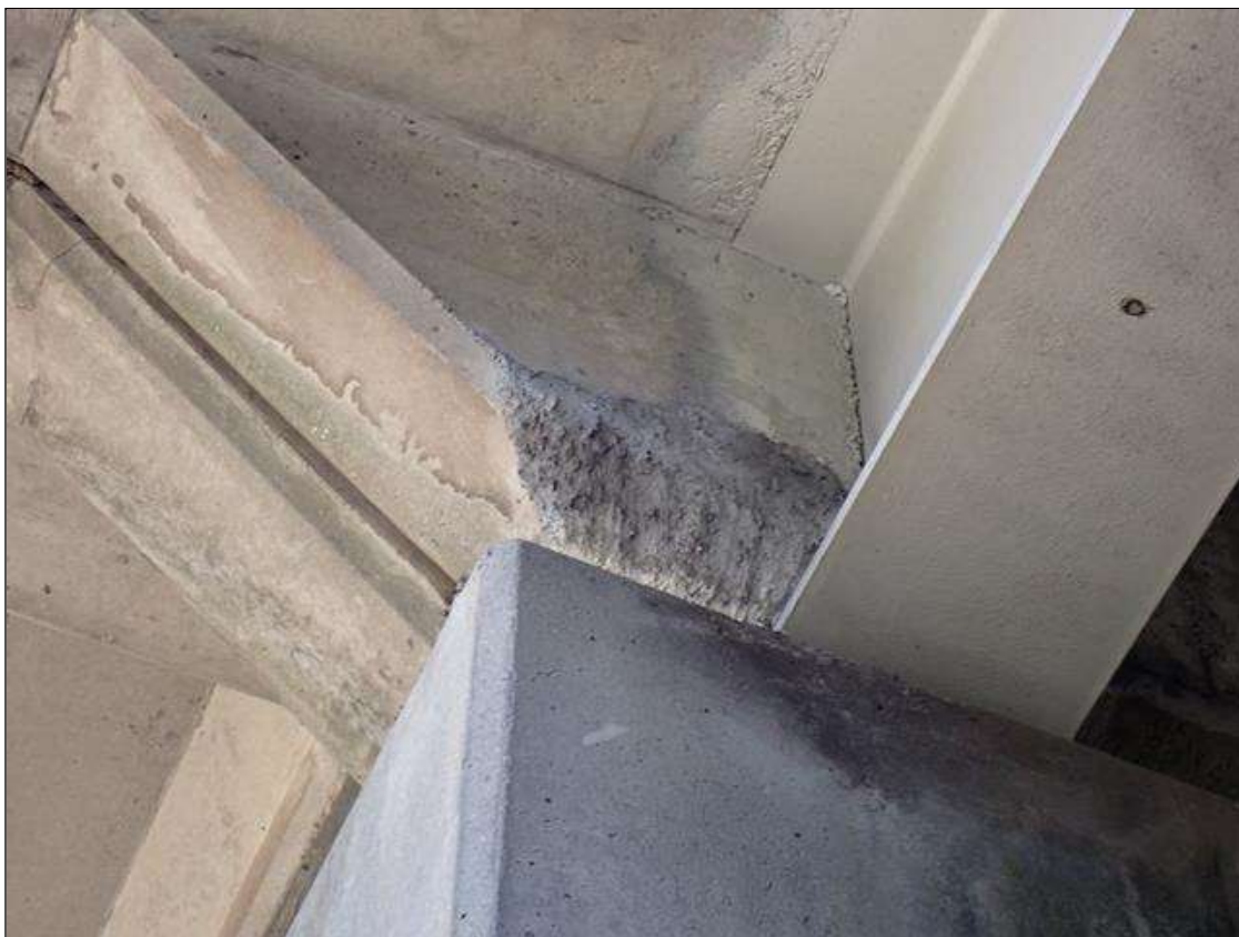
Span 2 Beam 1: 12 inch x 5 inch x 1.5 inch deep patched spall in end diaphragm, in west overhang at bent 2
