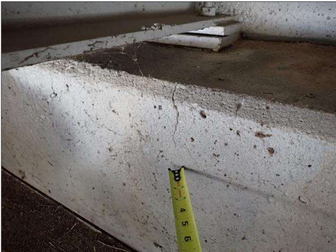
End Bent 2 Cap 1: 10 - vertical cracks up to 1/32 inch wide, in face of cap, at random throughout
