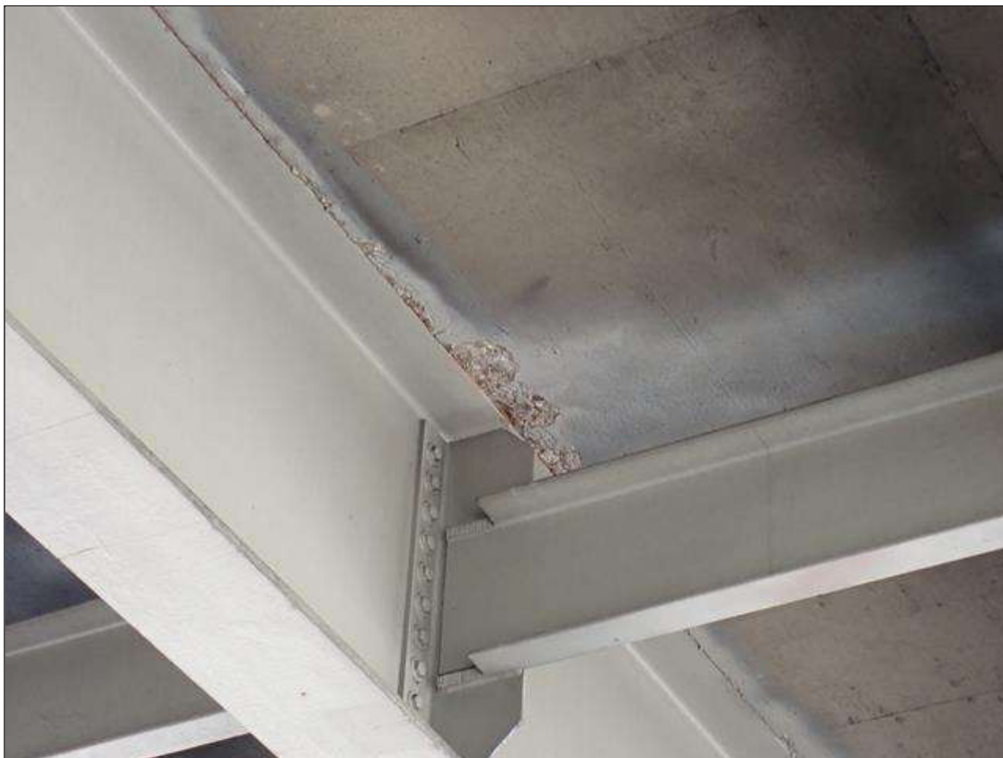
Span 3 Deck: surface spalling up to 1 foot x 4 inch x 1/2 inch deep, full length, underside of deck along both sides of beam 2.
