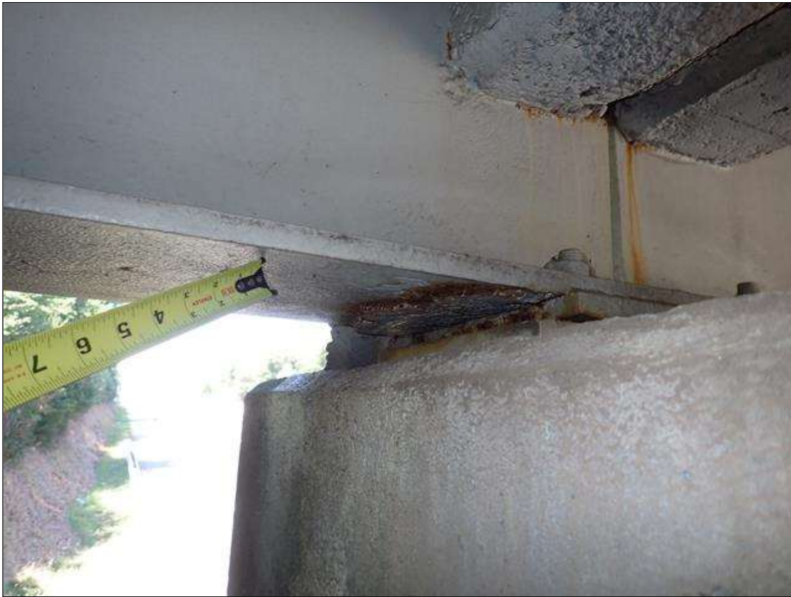
Span 1 Beam 1: (PAR) at bent 1, web adjacent to diaphragm, painted over section loss (3/8 inch average remaining x 3 inch x 2 inch); painted over pitting: lower web (up to 1/8 inch deep x 1 foot x 1 foot); bottom flange (up to 1/8 inch deep x 1 foot); underside of bottom flange, rust scale
