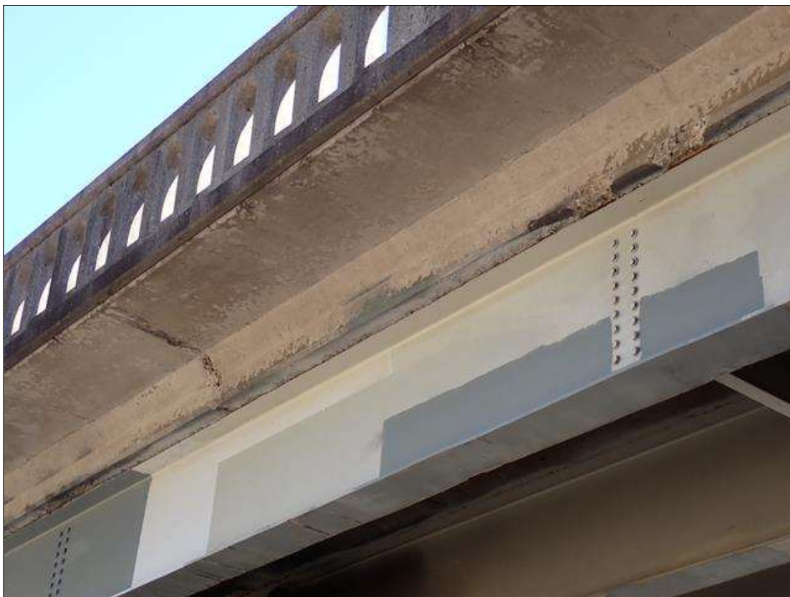
Span 3 Deck: spalling up to 12 INCH WIDE X 1 INCH deep, full length, underside of deck along both sides of beam 1.
