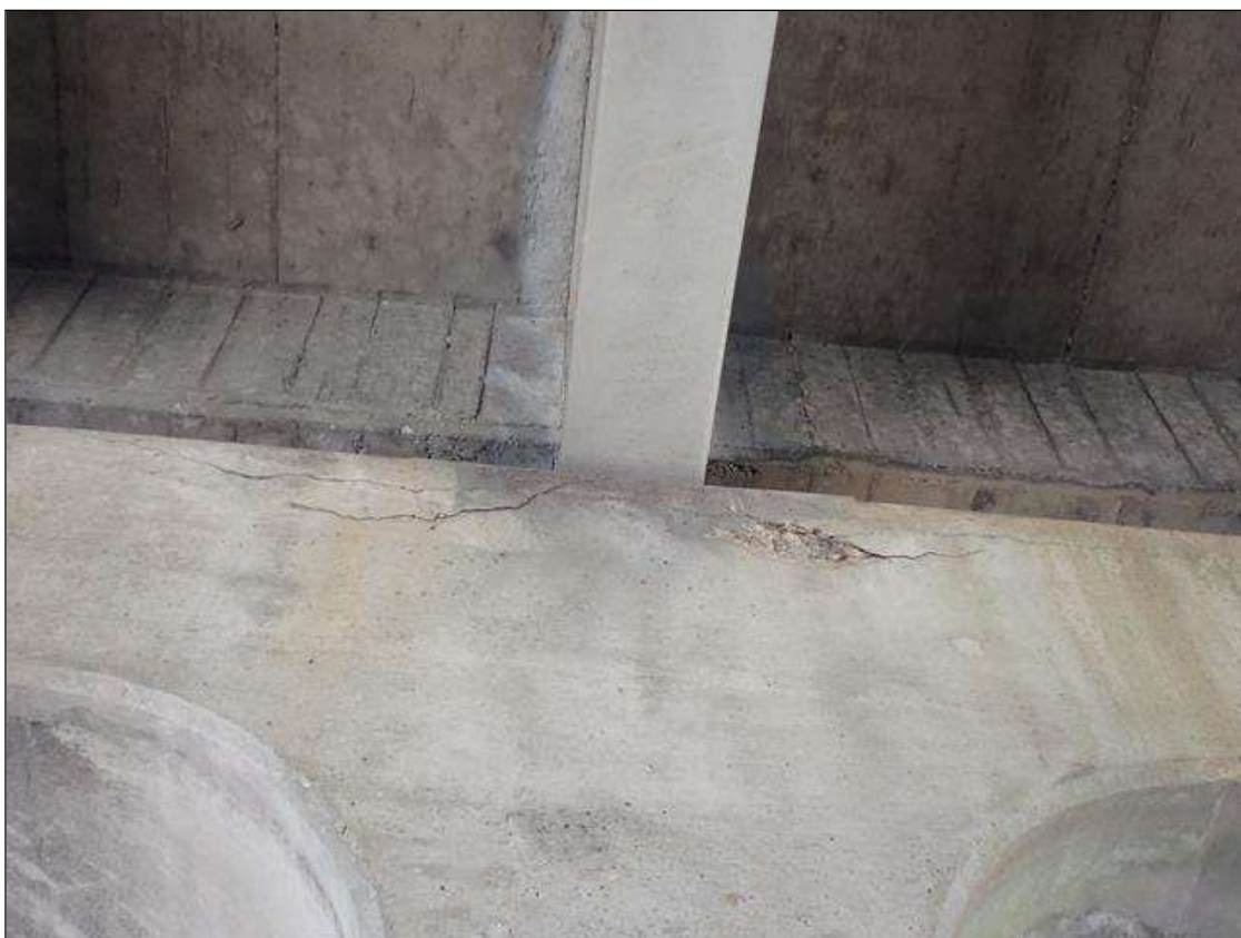
Bent 2 Cap 1: north face, below bays 2 and 3, near beam 3, spall/delamination (6 feet x 15 inch x up to 2 inches deep) with associated cracks (up to 1/16 inch)
