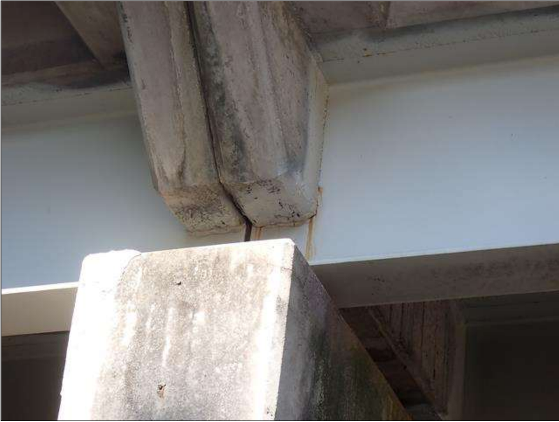
Span 2 Beam 5: (PAR) at bent 1, web adjacent to diaphragm, painted over section loss (approximately 3/8 inch average remaining x 7 inch x 1 inch); no safe ladder access to exterior face
