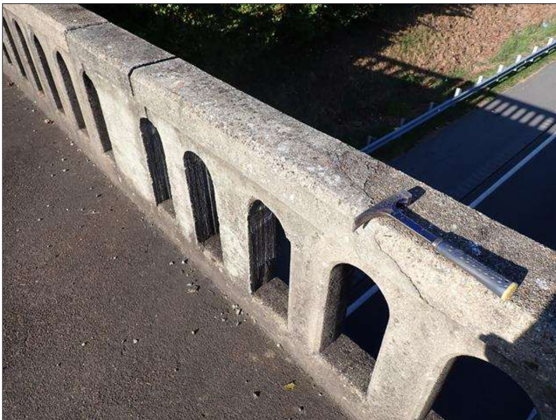
Span 2 Left Bridge Rail: 4 feet of patched rail and curb x full height, with cracks up to 1/32 inch, near midspan.
