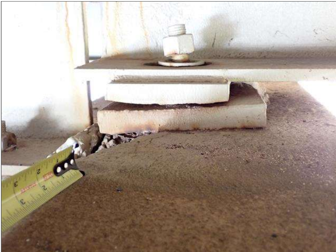
Span 4 Beam 3 - Near Bearing 3: (PAR) south edge of masonry plate, undermined (13 inch x 3 inches deep) due to cap step spall; masonry plate displaced downward (up to 1/2 inch)
