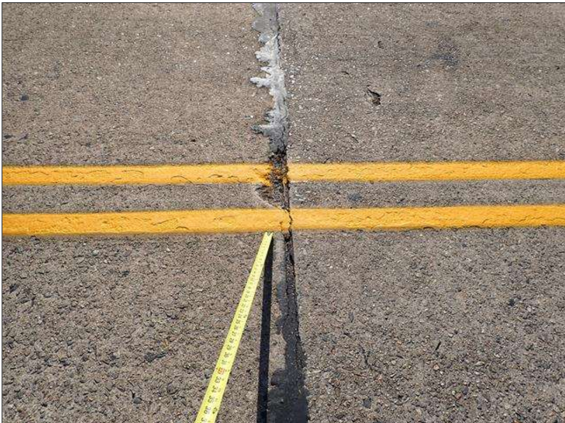
Span 4 Expansion Joint at Bent 3: missing joint material [up to full depth] in left and right shoulder, and centerline
