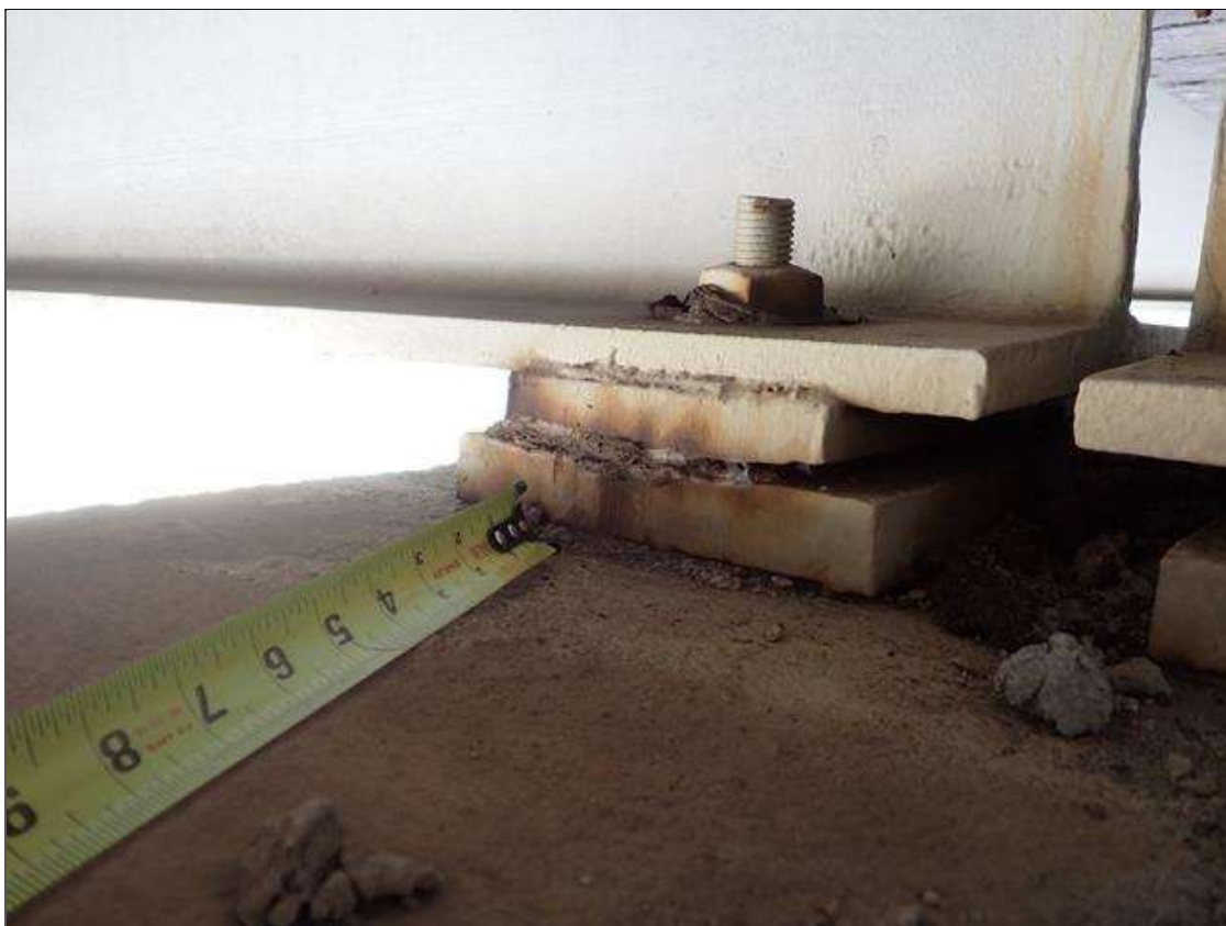
Span 3 Beam 3 - Near Bearing 3: surface rust/pack rust.
