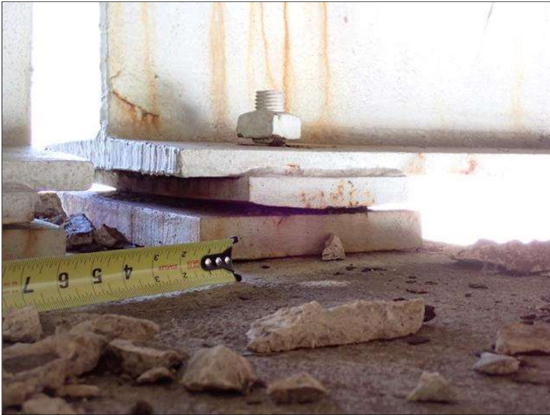
Span 3 Beam 1 - Near Bearing 1: freckled rust/pack rust
