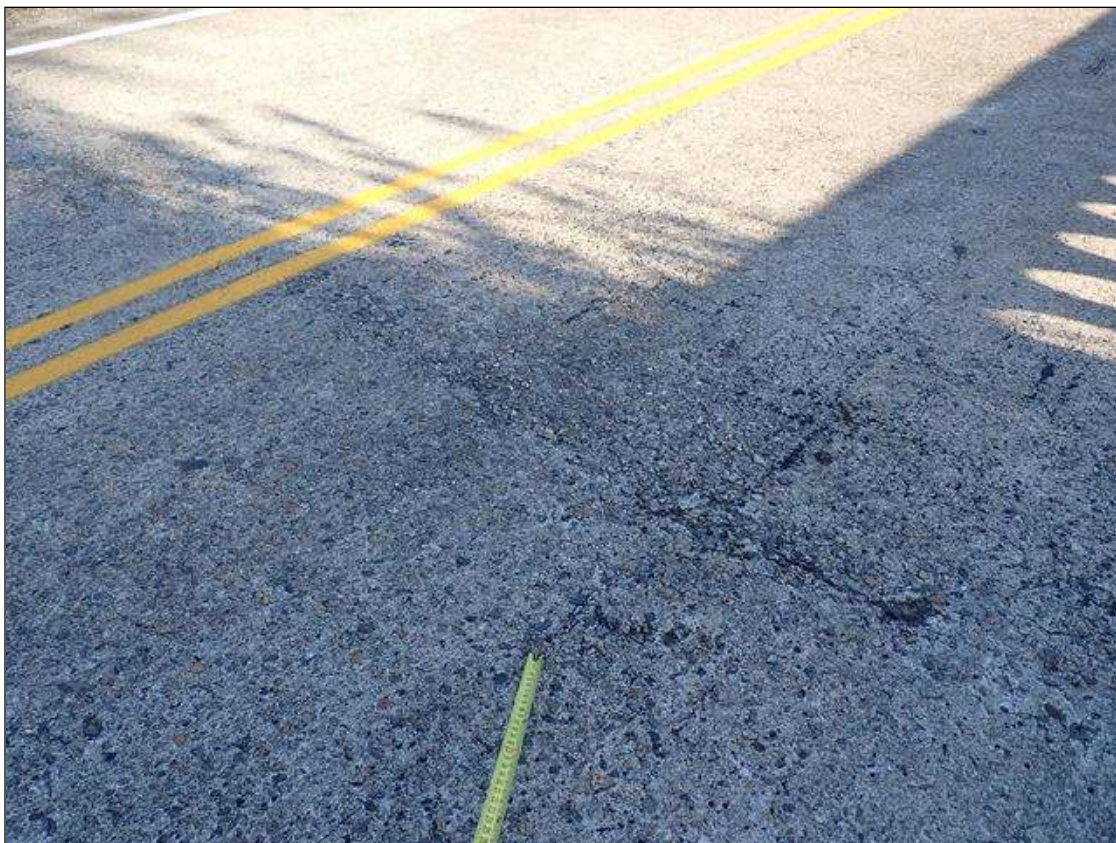
Span 1 Deck: throughout top of deck, wear with secure aggregate (up to 1/2 inch deep)
