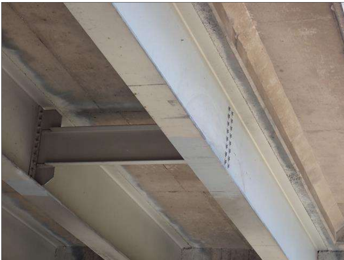
Span 3 Beam 5: 2023 area repainted with new impact scrapes; previously noted as: SUPPLEMENTAL INSPECTION IMPACT DAMAGE 2022.: two 1/4 inch deep indentations in bottom flange of beam 5 span 3 at 16.5 feet from bent 3 . SCATTERED SCRAPES
