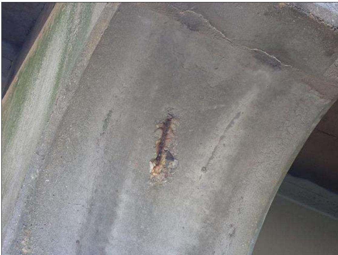
Bent 1 Cap 1: 10 inch x 2 inch x 1/2 inch deep spall with exposed reinforcing [no section loss noted] in West face underside of corbel
