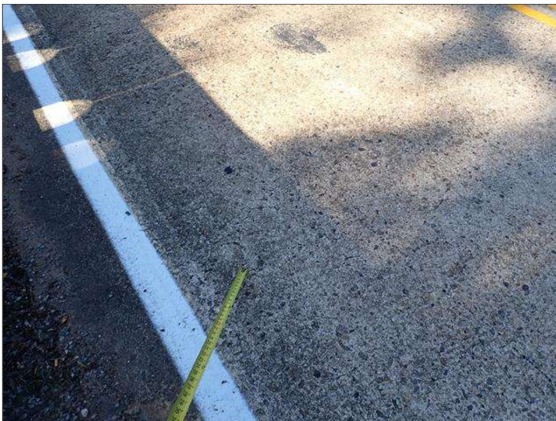
Span 4 Deck: random hairline map cracking and transverse cracks up to 1/32 inch wide on topside and underside.
