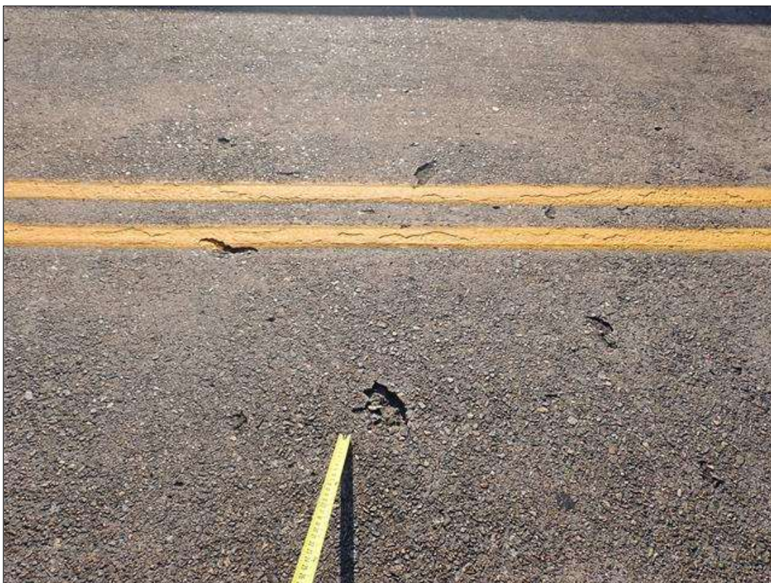
Span 2 Deck: throughout top of deck, spalls/delaminations (up to 6 inch diameter x 1 inch deep)
