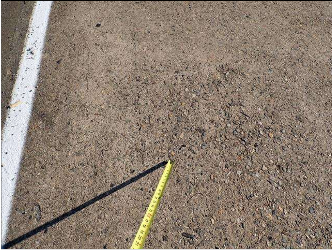
Span 3 Deck: random hairline map cracking and transverse cracks up to 1/32 inch wide.
