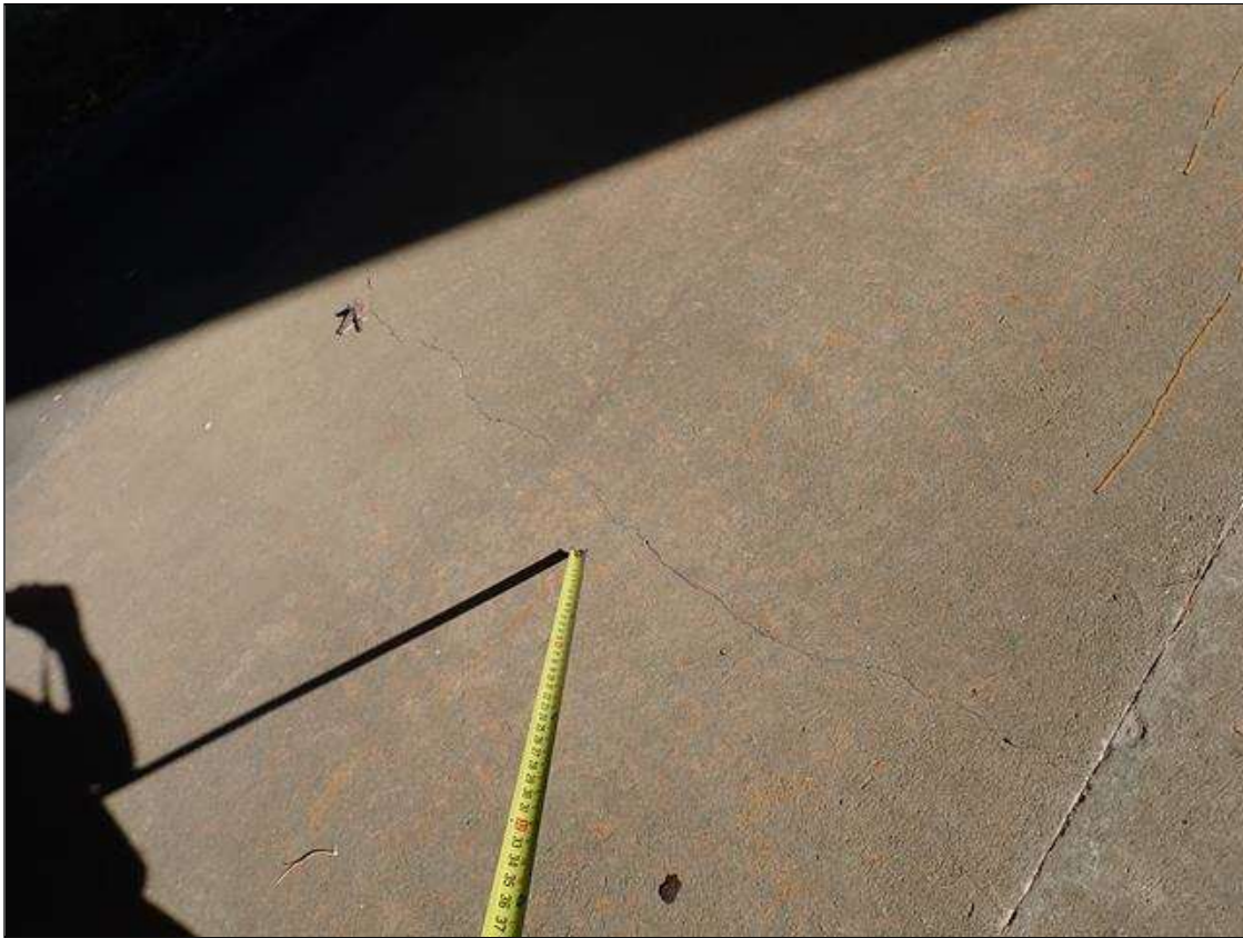
end bent 2 slope protection, at random, transverse cracks (up to 1/16 inch x 8 feet)
