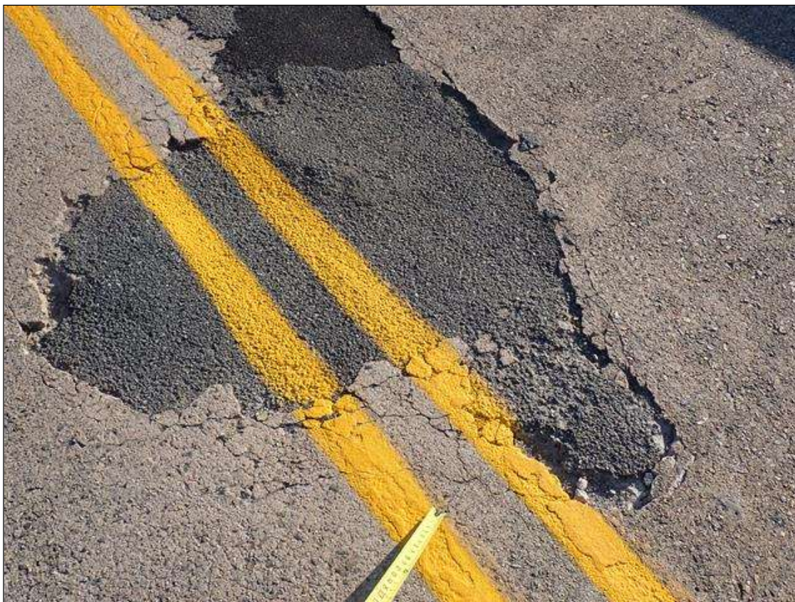
Span 2 Deck: up to 9 foot x 4.5 foot wide patches with up to 3 foot x 15 inch x 1.5 inch deep spalls/delaminations, at centerline, far half of span.
