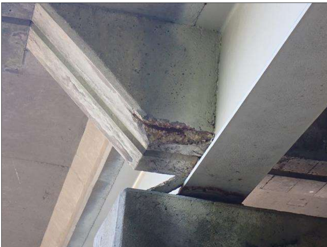
Span 1 Beam 1: 15 inch x 6 inch x 1.5 inch deep spall with exposed reinforcing, in end diaphragm, west overhang, at bent 1.
