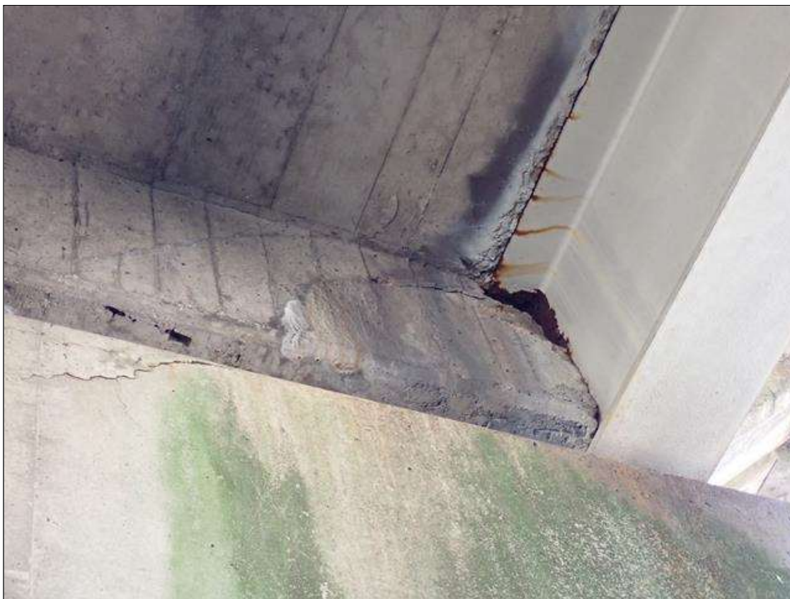
Span 3 Beam 1: bay 1 end diaphragm at bent 2, spall (1 foot diameter x 2 inch deep) with adjacent diagonal crack (1/32 inch x 3 feet) with efflorescence
