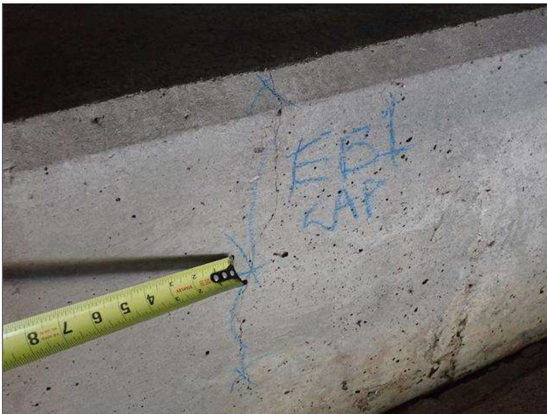
End Bent 1 Cap 1: 10 - vertical cracks in North face extending to topside of cap up to full height x 1/32 inch wide, at random throughout
