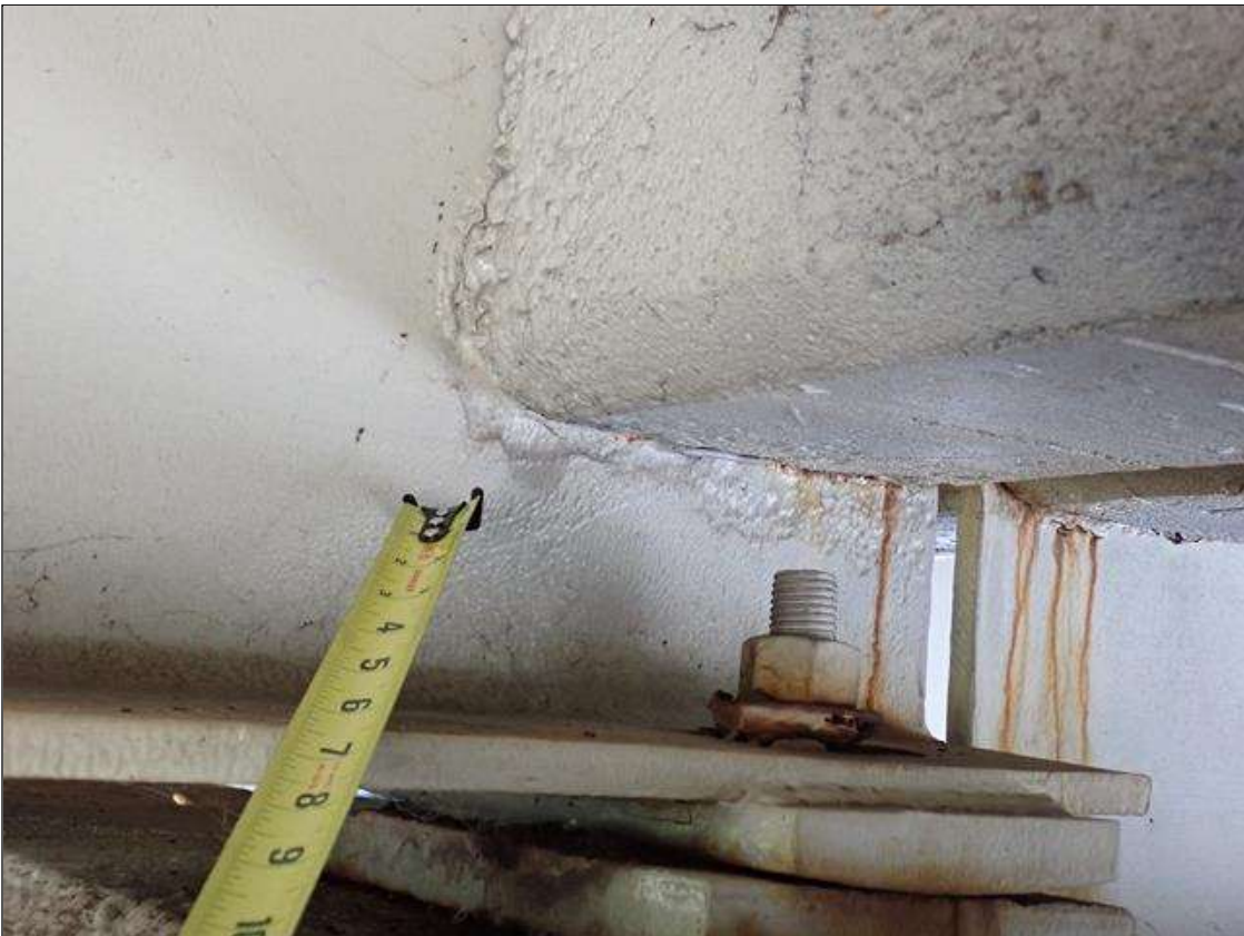
Span 4 Beam 3: (PAR) at bent 3, web adjacent to diaphragm, painted over section loss (1/4 inch average remaining x 12 inch x 4 inch)
