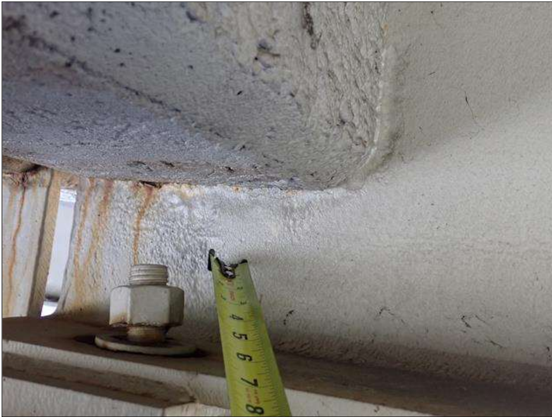
Span 4 Beam 3: (PAR) at bent 3, web adjacent to diaphragm, painted over section loss (1/4 inch average remaining x 12 inch x 4 inch)
