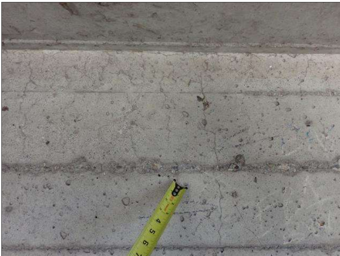
End Bent 1 Abutment: throughout backwall in all bays, multiple areas of hairline map cracking
