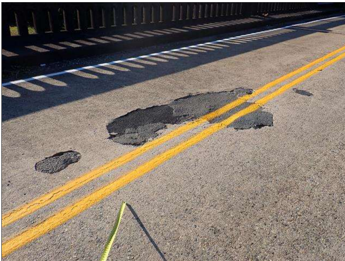
Span 2 Deck: up to 9 foot x 4.5 foot wide patches with up to 3 foot x 15 inch x 1.5 inch deep spalls/delaminations, at centerline, far half of span.
